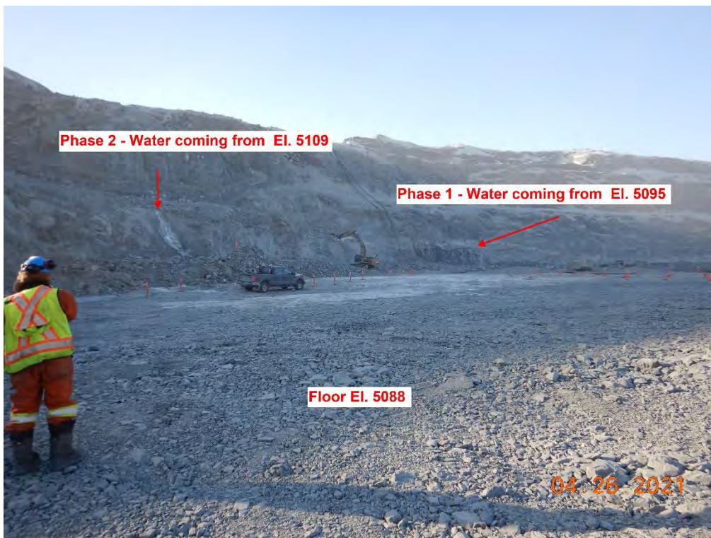
Photo 4: Pit seepage along south wall, looking southeast (April 26, 2021).
