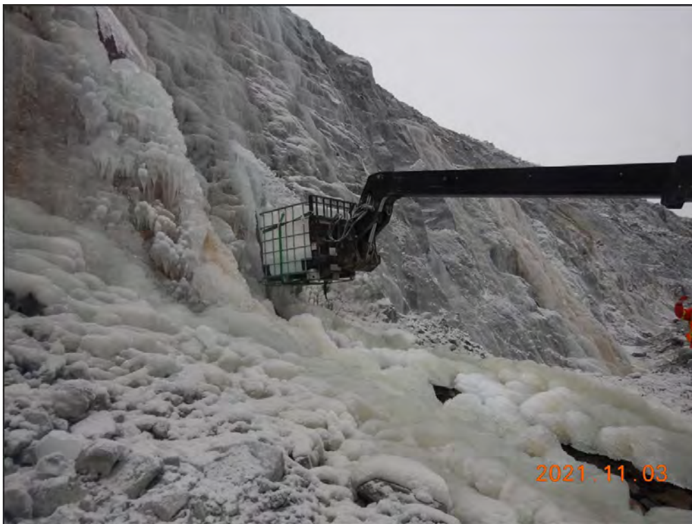
Photo 8: Pit seepage along south wall, looking southeast towards Drill hole-1 during flow measurement (November 2, 2021).
