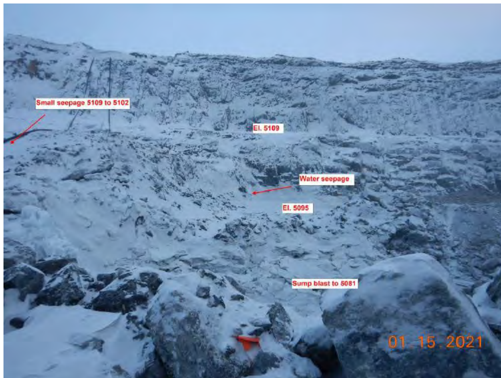
Photo 1: Pit seepage along Whale Tail Pit south wall, looking south (January 15, 2021).
