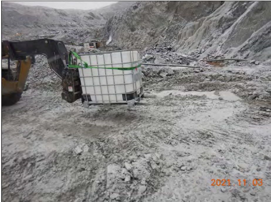
Photo 9: Pit seepage along south wall, looking northeast of Drill hole-1 and seepage sample location ST-GW-WT-1 (November 2, 2021).
