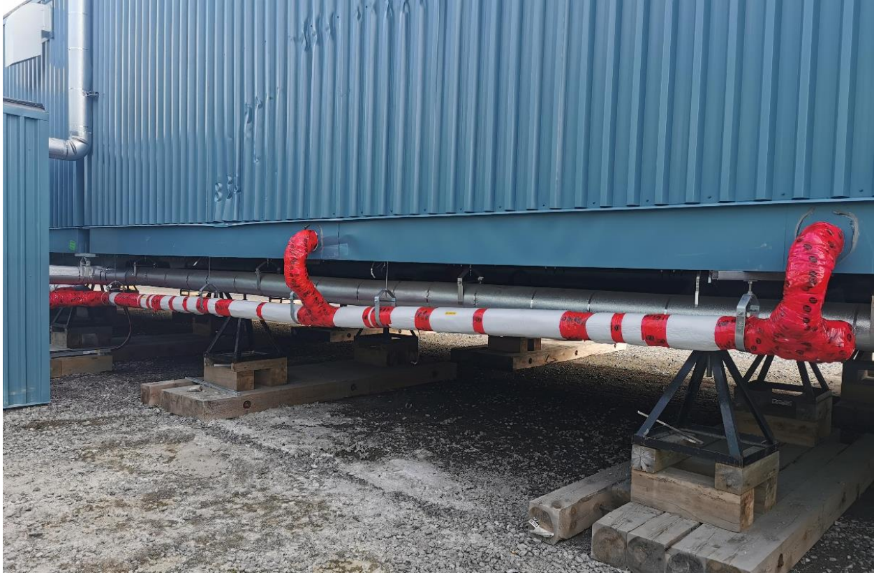
Figure 4: Clean up of the area and reinstallation of the drainpipe with heat trace and insulation.
