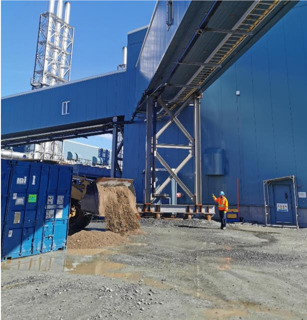
Figure 2: Sand berm being created at the south end of the spill location to contain the heat recovery water.
