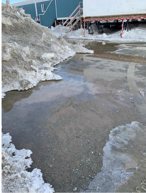
Figure 4: Water pooling on south side of the main camp.
