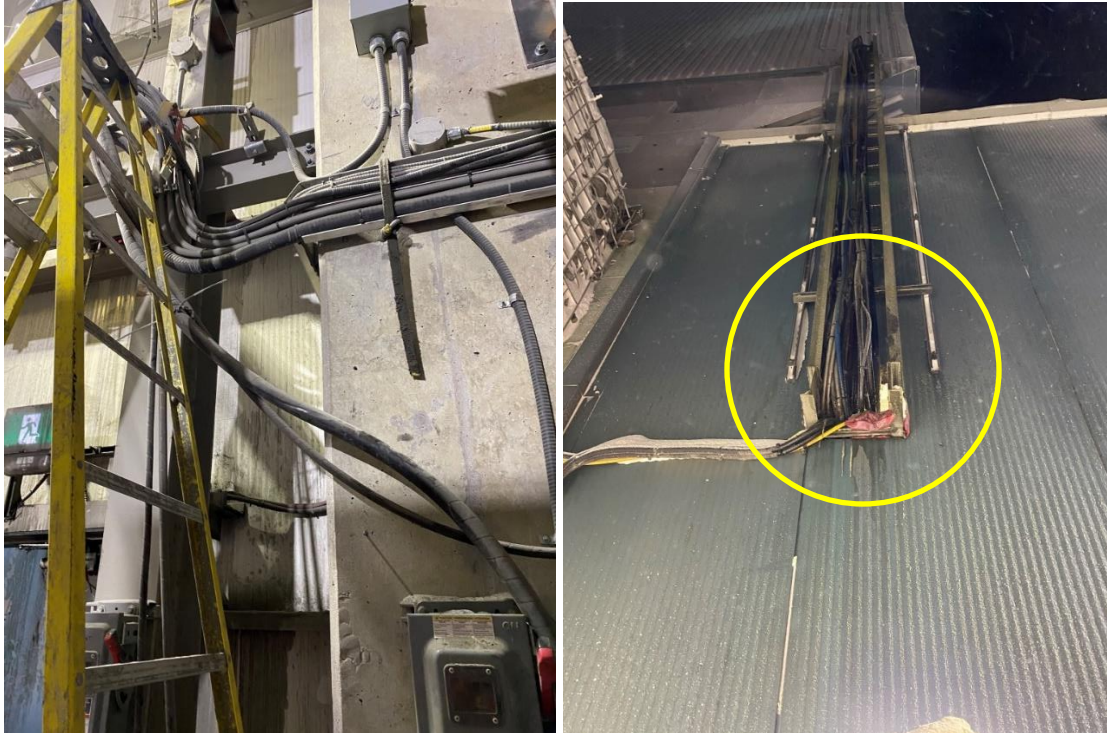
Figure 2: A hydraulic line breakage occurred on the exterior of the building (circled area).
