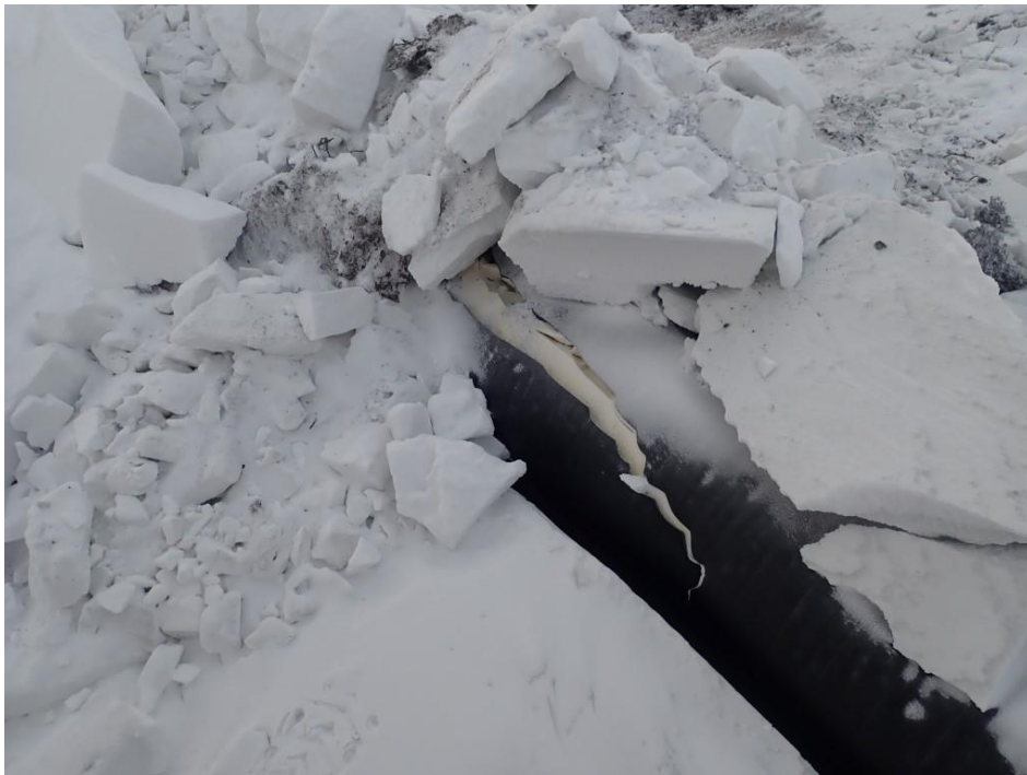
Figure 3: Damage to heat recovery waterline.
