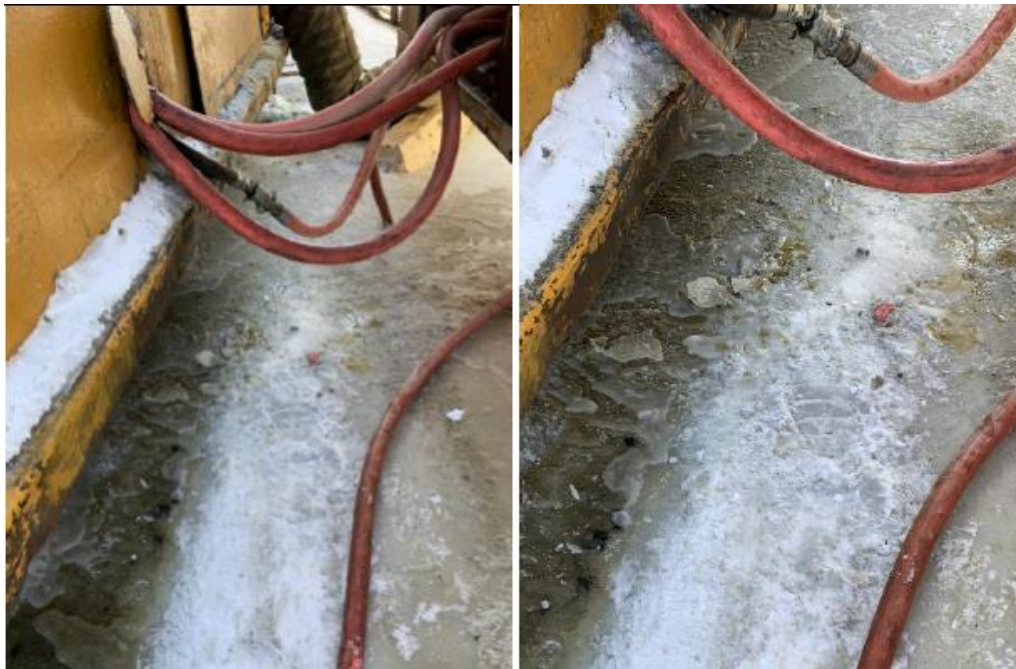
Figure 3: Hydraulic oil dripping from hoses outside of Drill #7.
