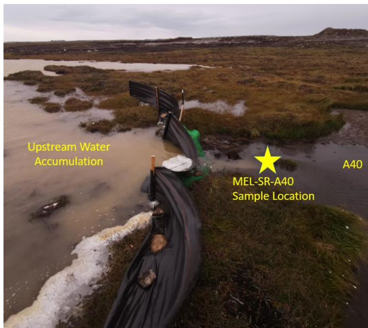
Figure 2: Installation of sediment control fence and logs. Sample location established immediately downstream of the sediment control fence.
