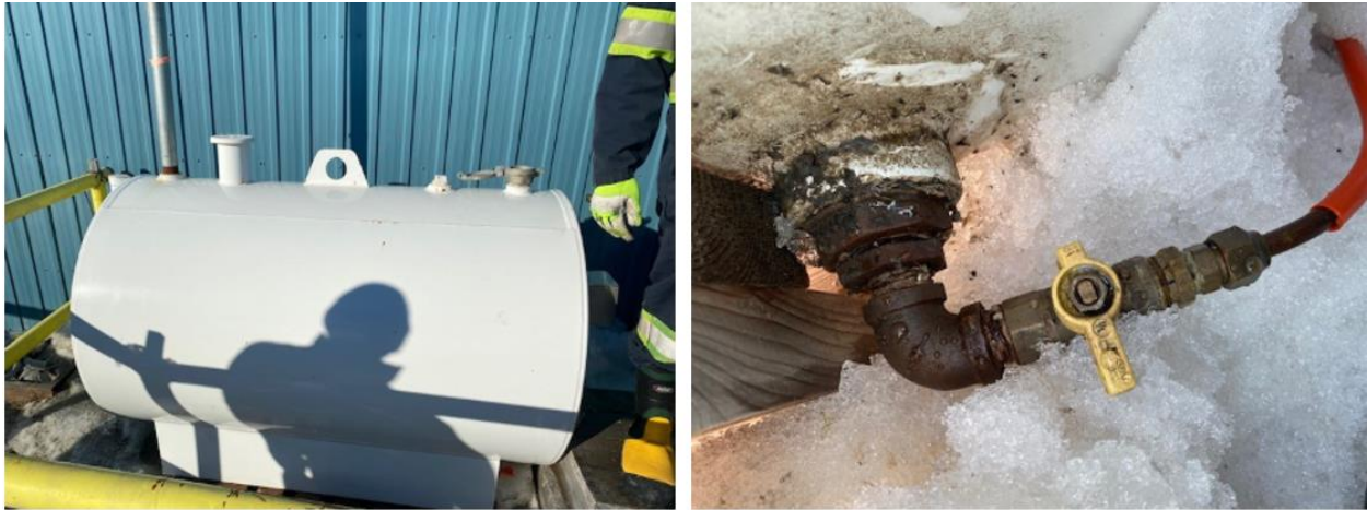
Figure 2: The exterior fuel tank and damaged fuel line which led to the spill.
