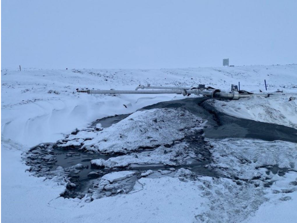
Figure 2: Cement paste leak
