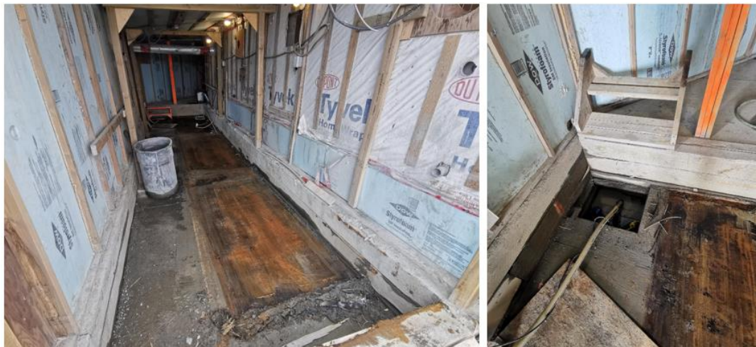
Figure 5: Decantation room cleared of all materials, and the down slope sump actively being pumped of standing diesel.
