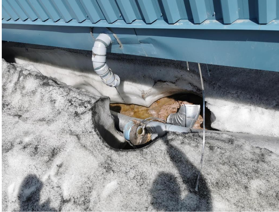
Figure 2: Drainpipe on the exterior of Wing 12 that separated from the building due to the weight of snow.
