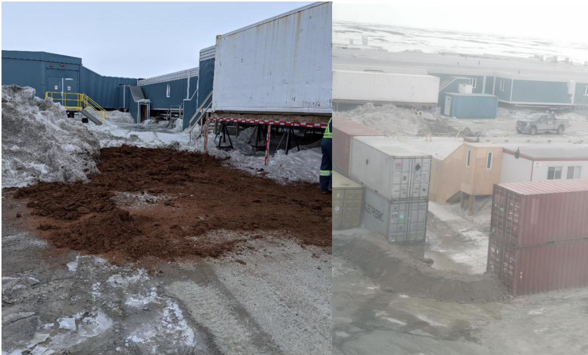
Figure 6: Clean peat/soil was used to absorb pooling water, and a temporary berm construction to mitigate downstream flow.
