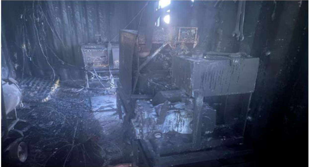
Figure 2: Photos of the pump shack after the fire was suppressed and the shack was towed back to the shop.
