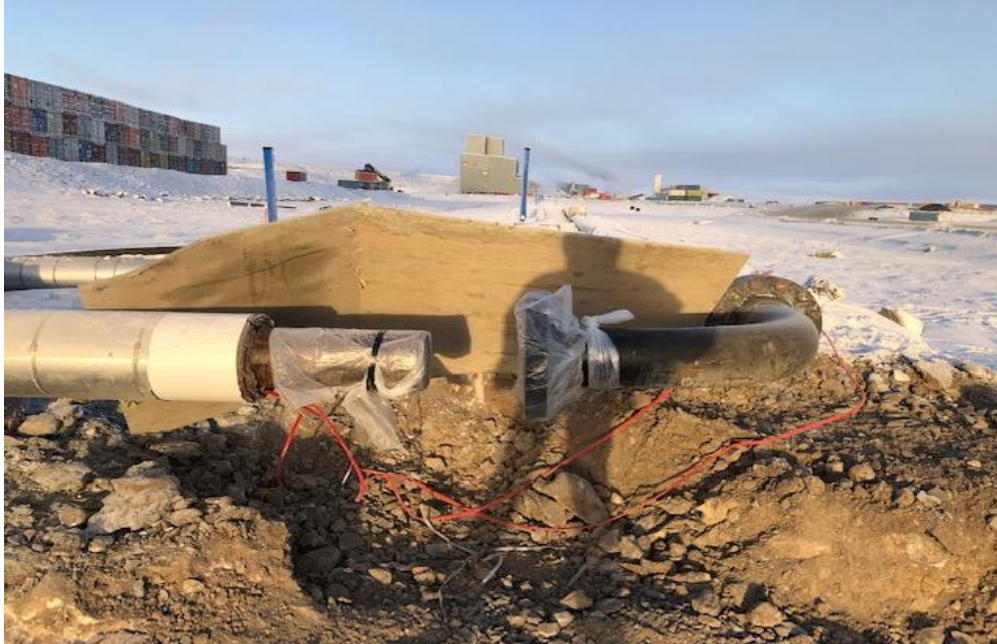
Figure 3: Disconnected line and remediated area
