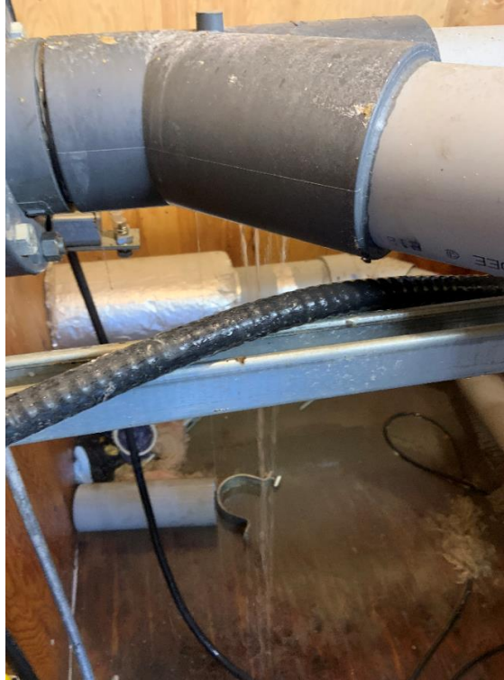
Figure 2: Cracked and leaking pipe joint inside the lift station.
