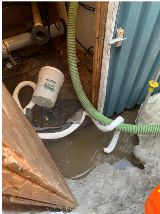
Figure 3: Entrance door of the lift station and water pooling directly outside.
