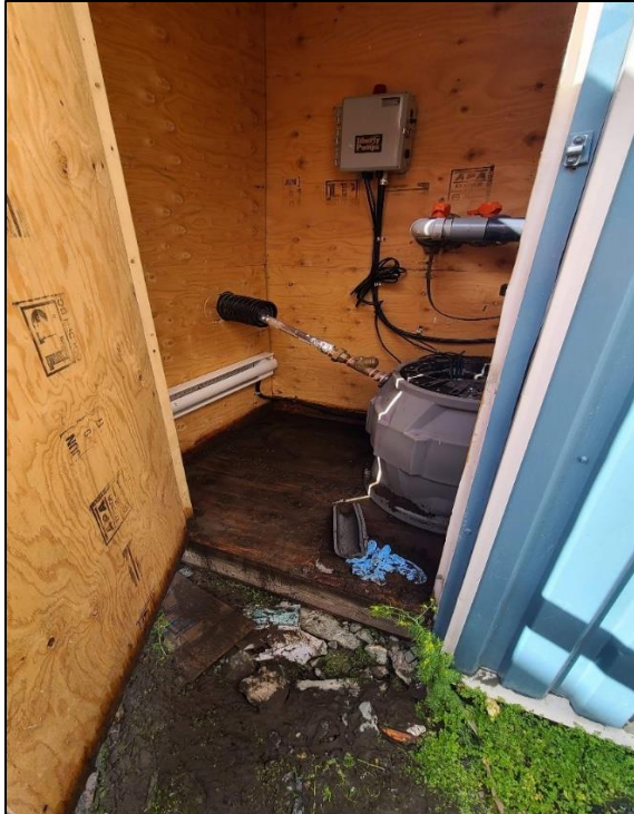
Photo 1: Wing-C lift station spill
