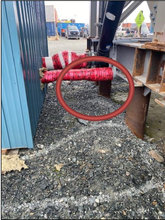
Photo 1: Sewage spill location
