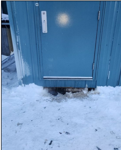
Photos 1: Sewage spill outside life station.
