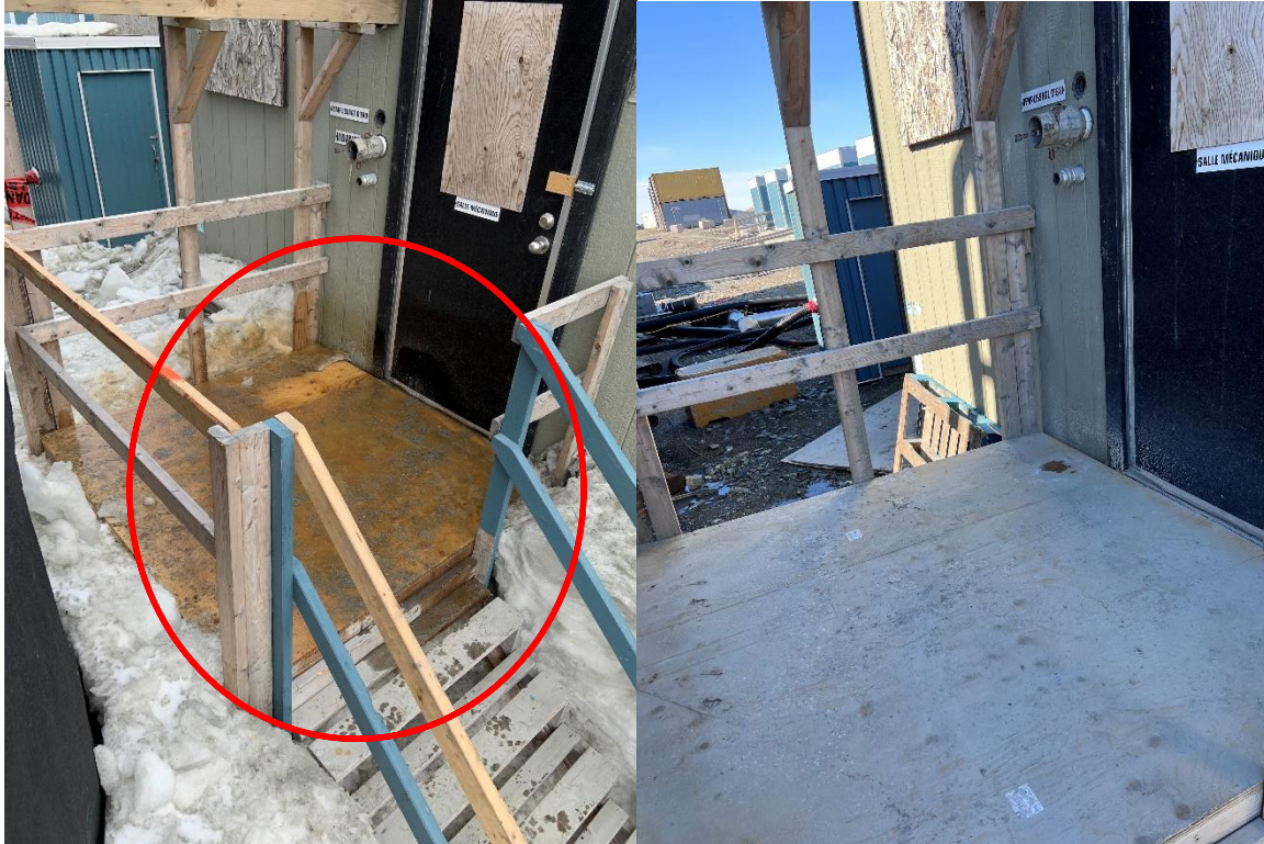
Figure 2: C wing lift station spill and cleanup
