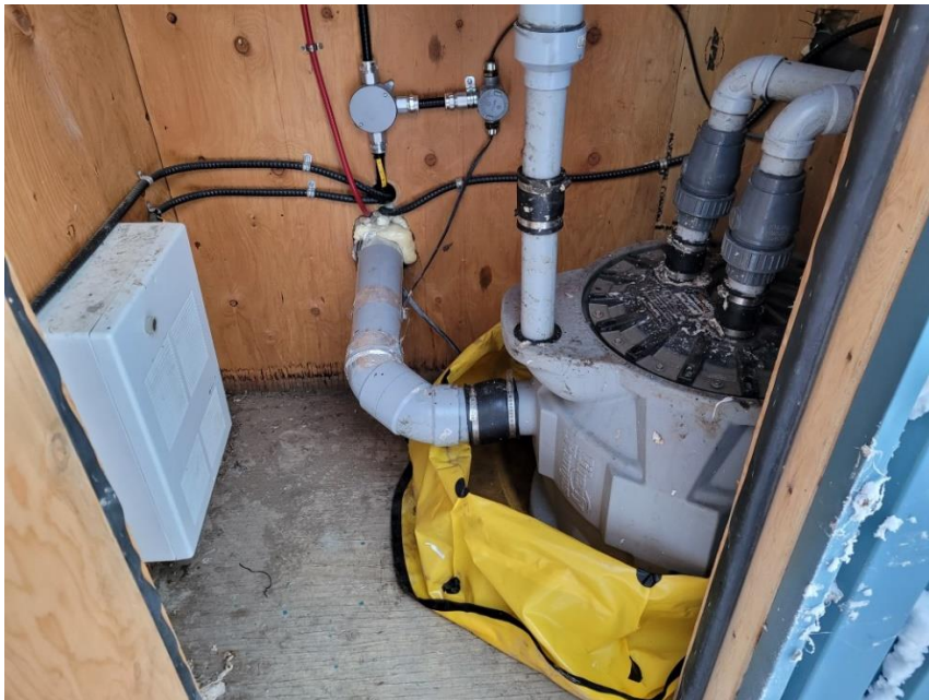
Photo 3: Wing three lift station with secondary containment installed post cleanup
