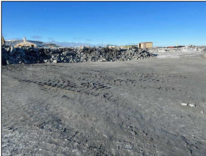
Photo 2: Hydraulic oil spill remediation area
