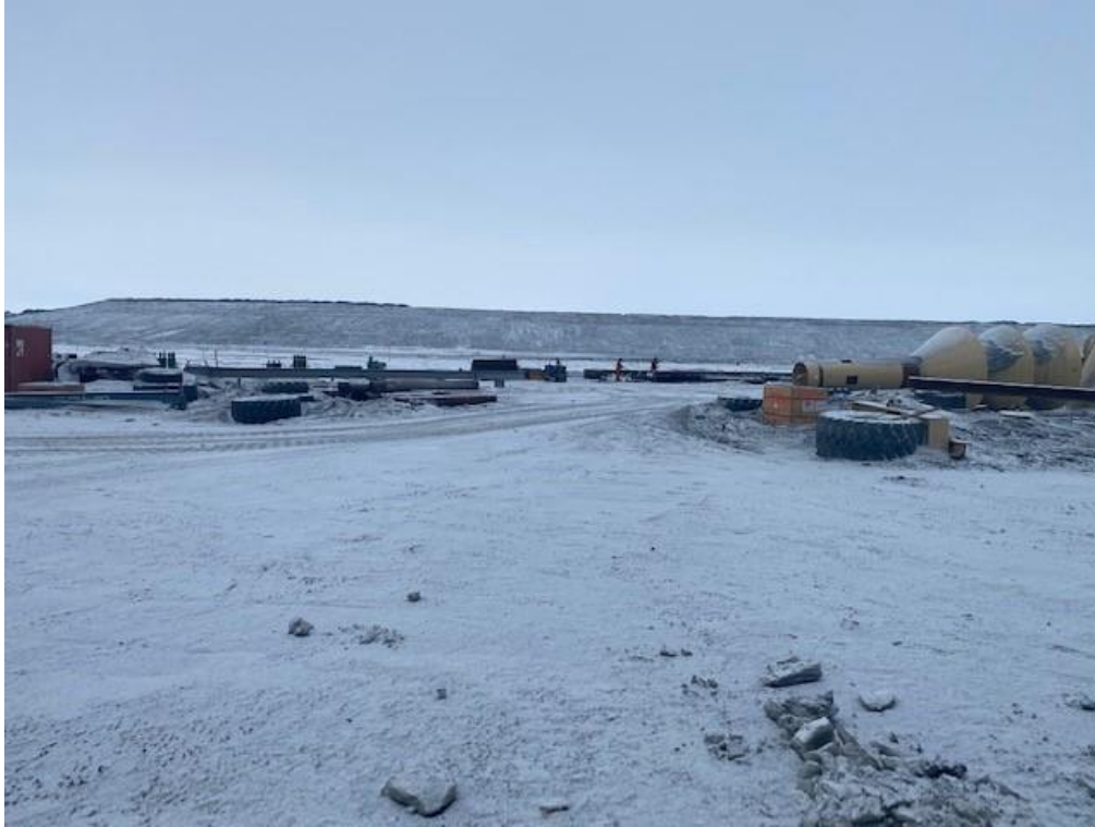
Figure 2: Thickener process water spill clean up
