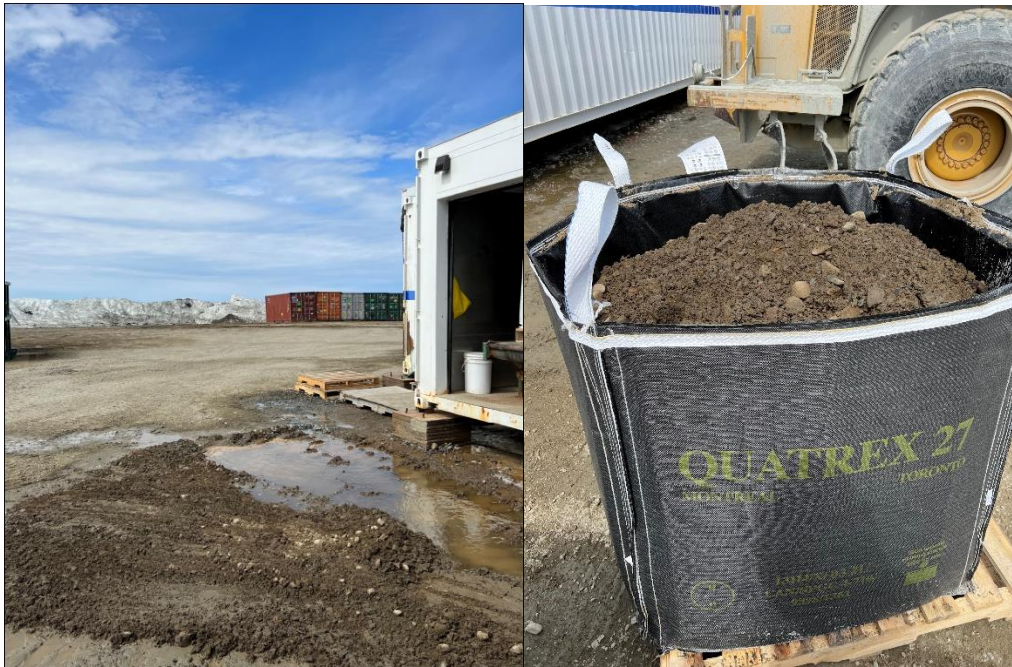
Figures 3-4: Spill area final cleanup and contaminated material packeted and ready to be disposed
