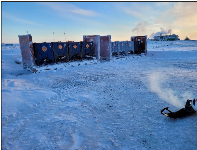
Photo 2: Emulsion spill remediation
