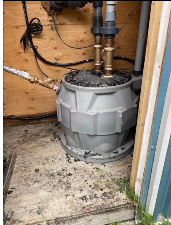
Photo 2: Wing C lift station spill remediation
