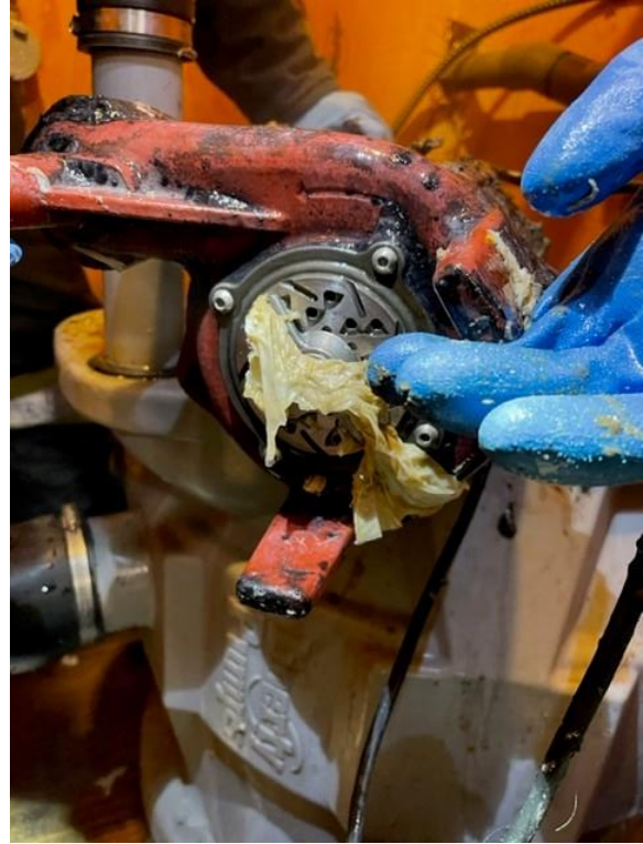
Photo 2: Wing three lift station grind pump blade
