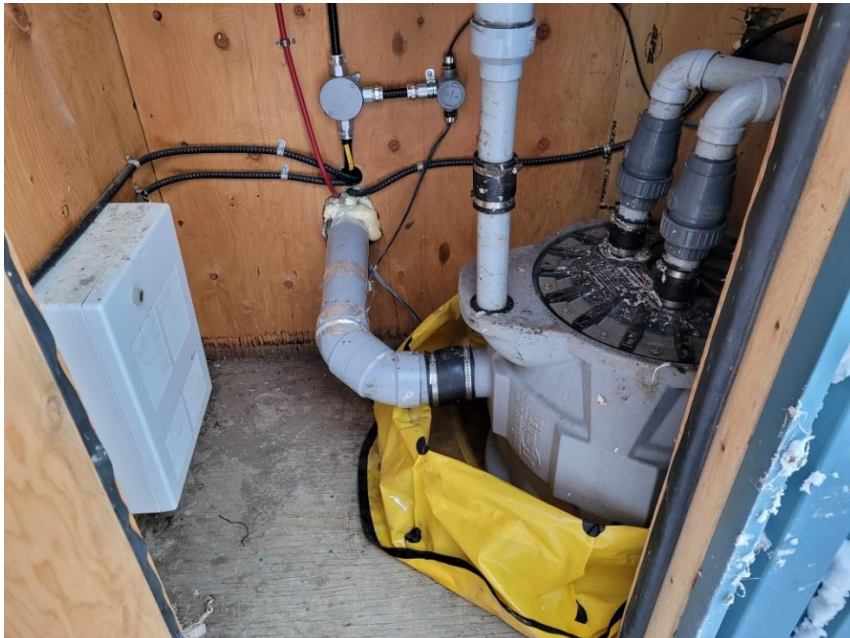
Photo 4: Wing three lift station with secondary containment installed.
