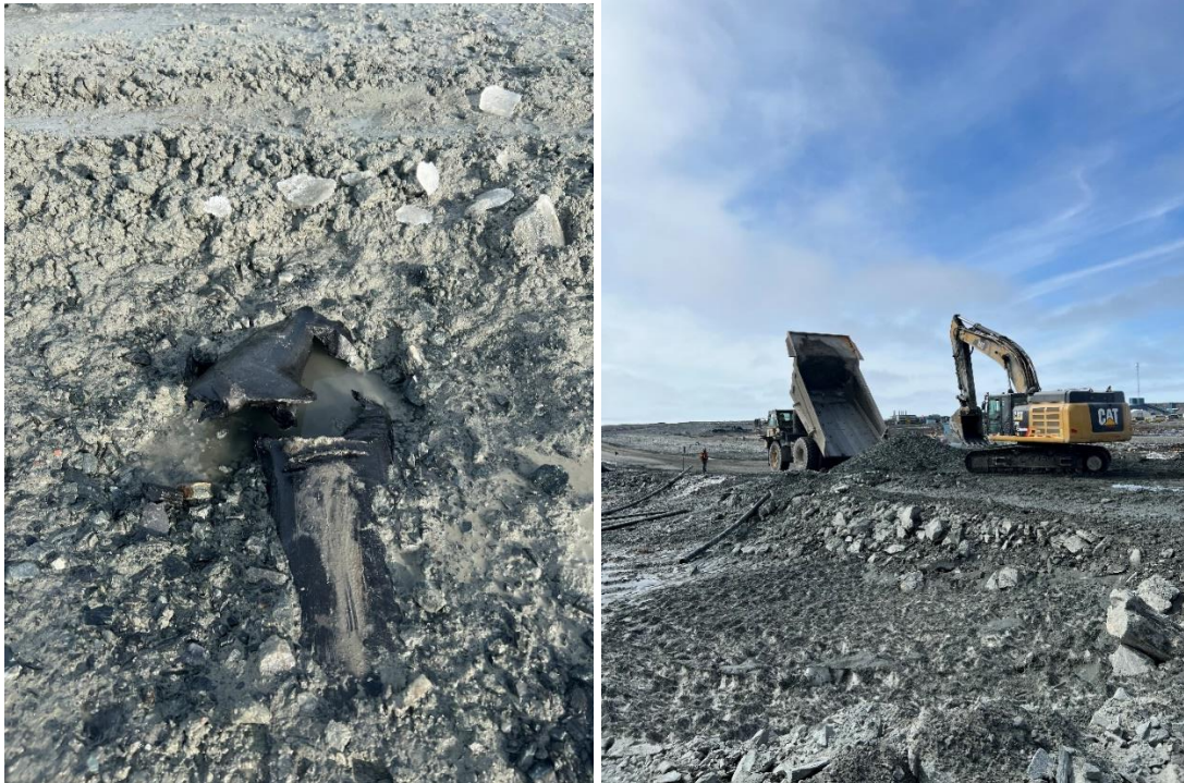
Figure 2 and 3: Damaged pipe which saline water flowed out of (left) and repairs made the same day (right).
