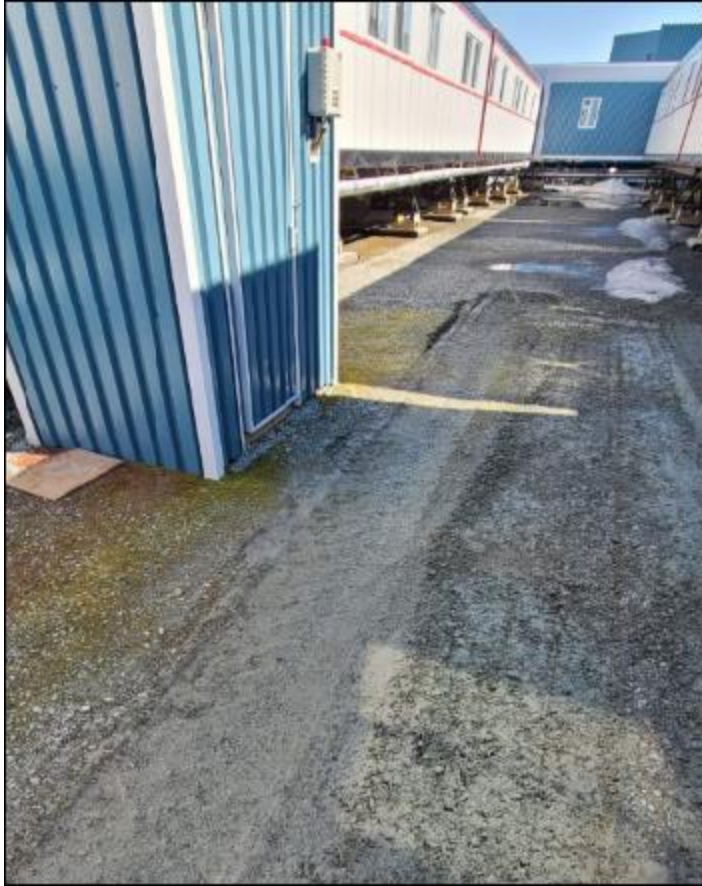
Figure 2: Location of sewage spill post-cleanup.
