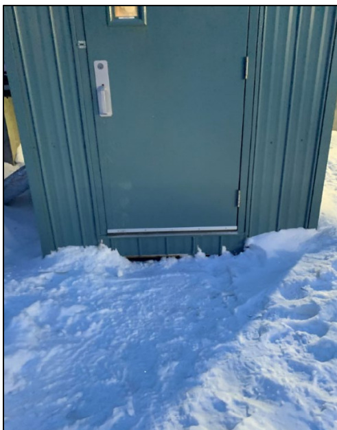
Photo 3: Sewage spill location post clean up.
