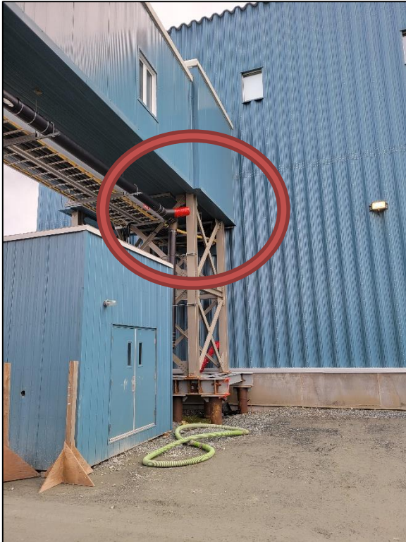
Photo 1: MSB remediated spill area.
