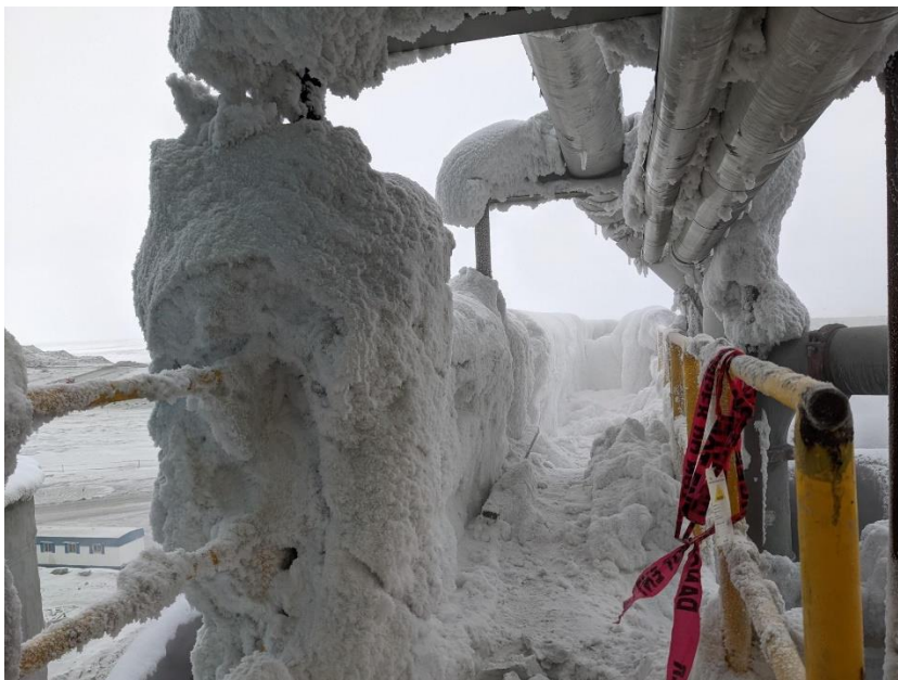
Figure 3: Pre-clean up of the overhead ice on the thickener tank (caused by humidity)
