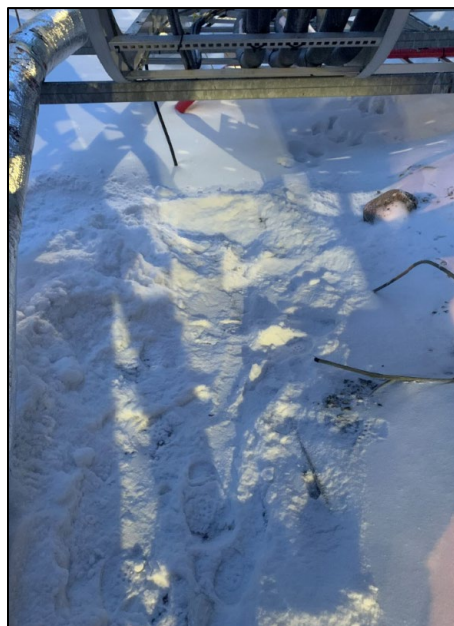
Photo 4: Sewage spill location post clean up.
