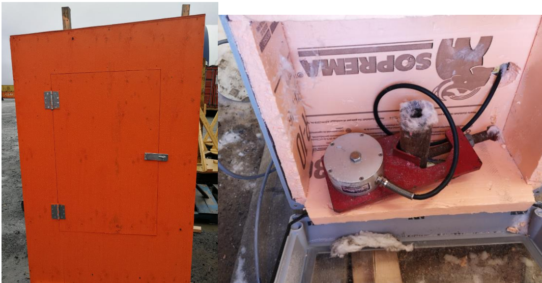
Figure 6. Surface Installation (Shelter & installation inside)
