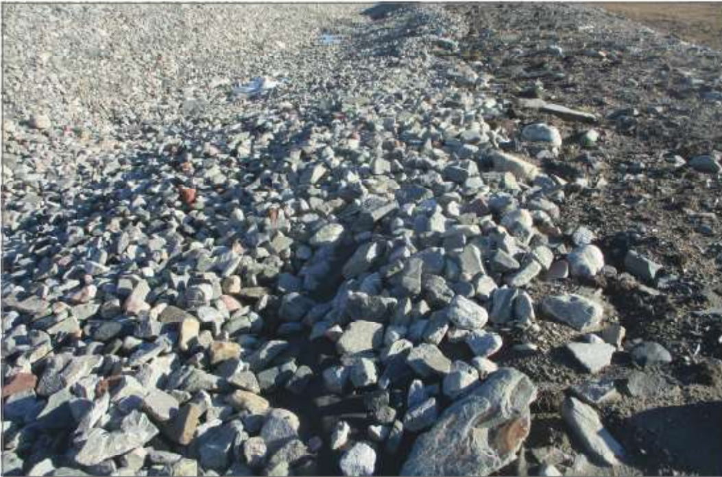
Photo 26: Channel 4 - Minor subsidence between original ground and channel rip rap.
