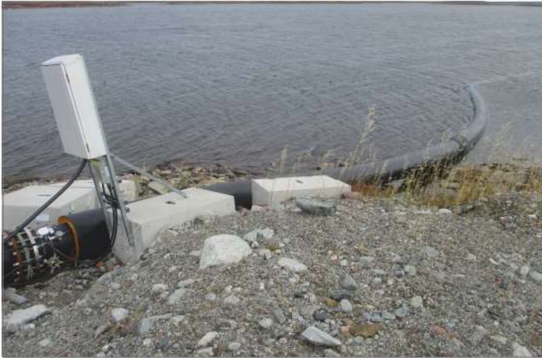
Photo 5: Exploration Camp—Diffuser line
