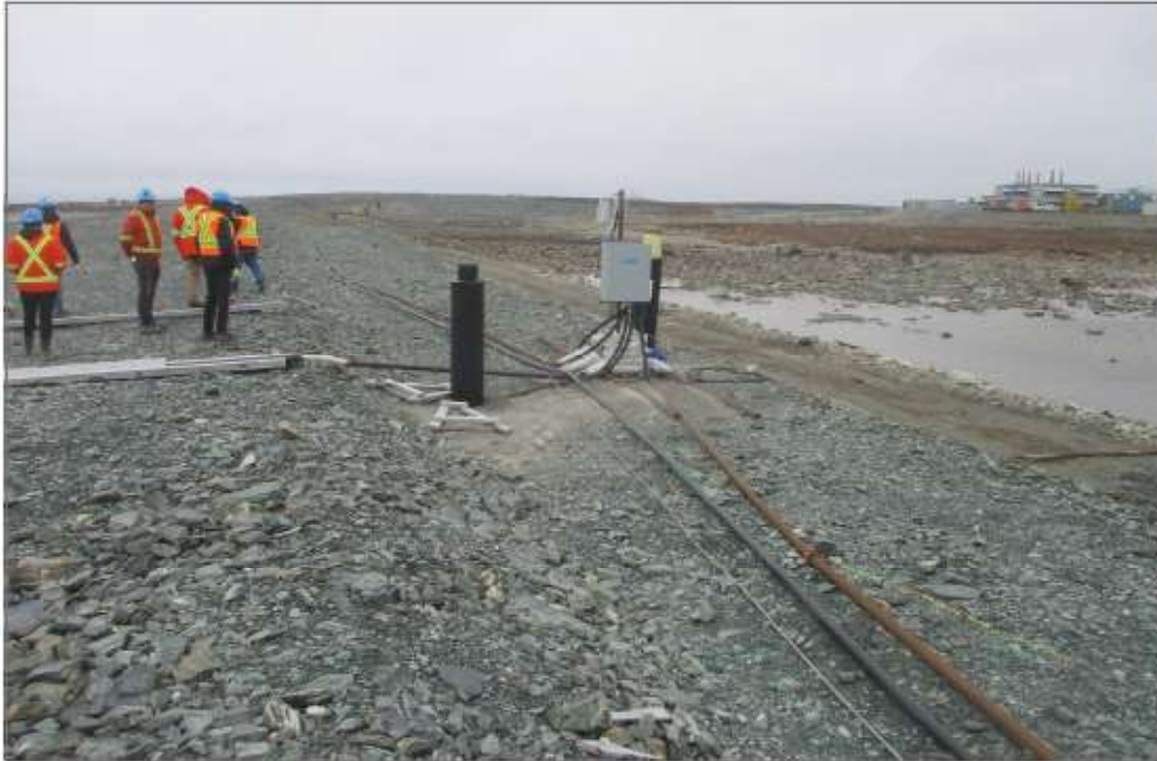
Photo 5: D-CP5 Dike - upstream, data logger, and GTC housings.
