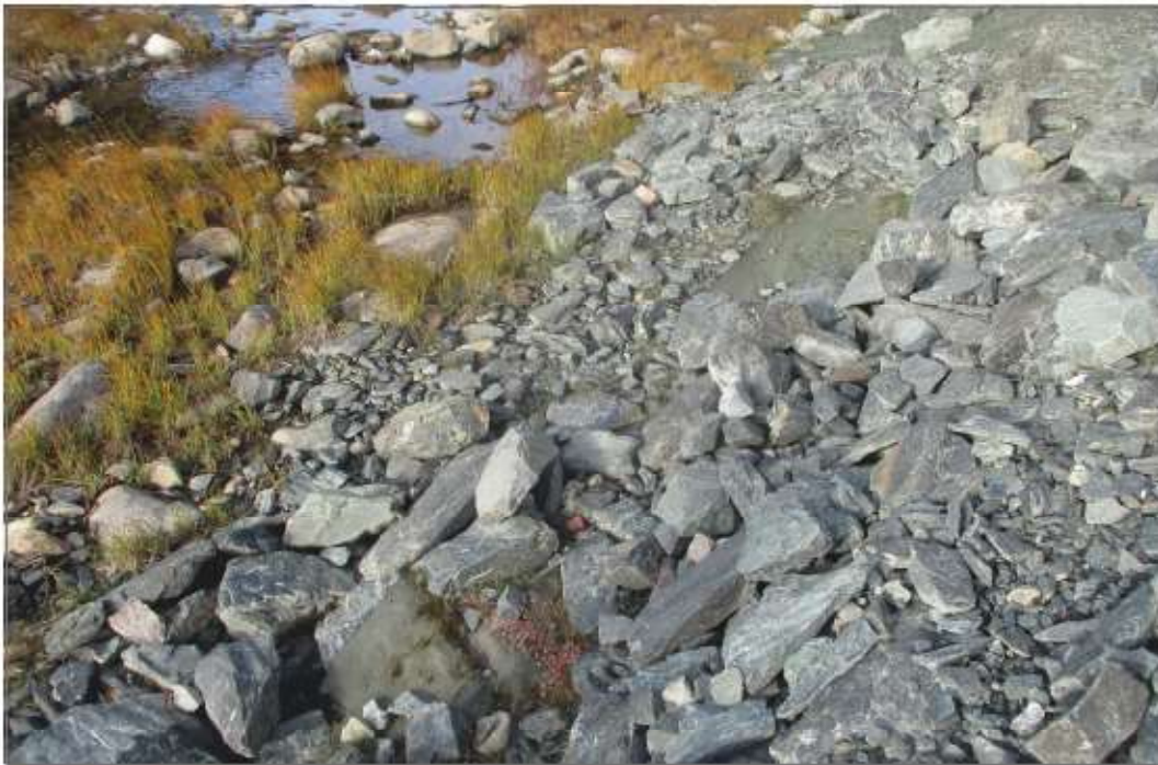
Photo 20: M-5 Bridge—Geotextile exposed at north abutment .
