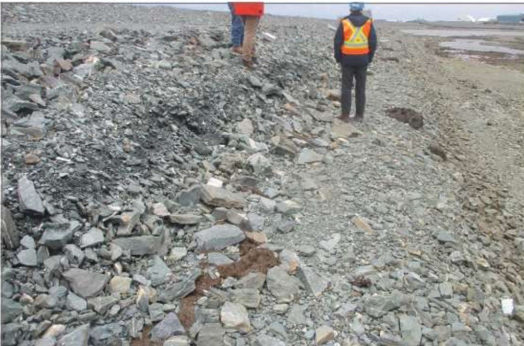
Photo 2: Dike D-CP1—Upstream face—some wave erosion evident, scarp approximately 1 m high. Erosion also evident on lower portion of slope. Slope is self armoured with larger particles in ROM fill.
