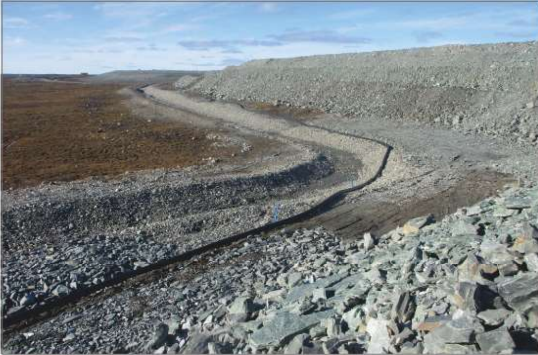
Photo 29: Channel 4 - Repaired rip rap slope and rockfill capping over preferential flow area between WRSF1 and Channel 4.
