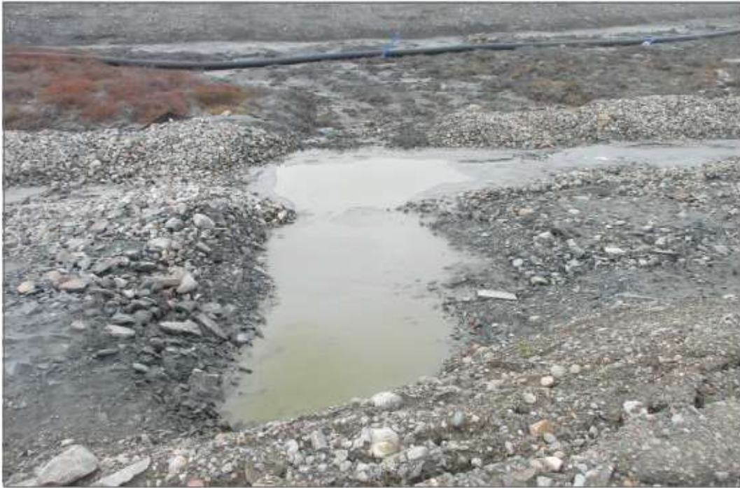
Photo 19: Channel 3—Subsidence across channel alignment, looking southeast.
