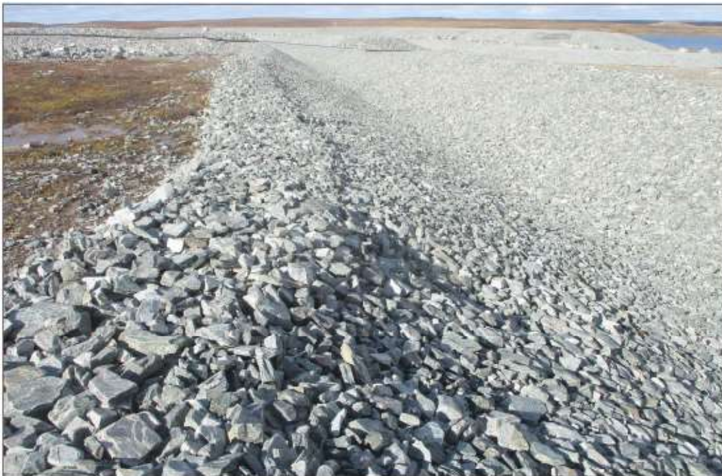
Photo 44: Channel 10—Slight subsidence of upstream slope and rip rap.
