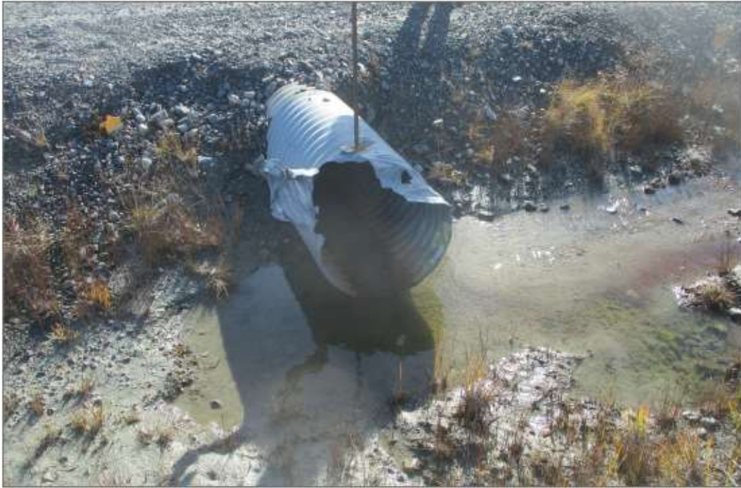
Photo 1: Culvert km 5.5—Damage to inlet.
