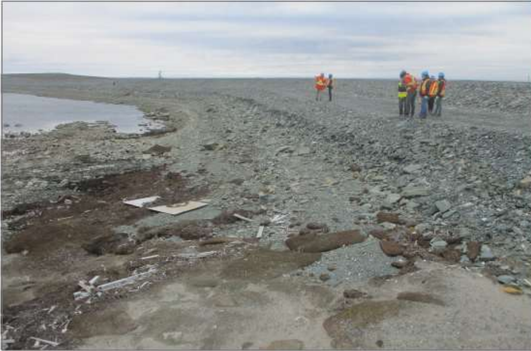
Photo 1: Dike D-CP1 - Upstream face—some wave erosion evident from 2019 event.
