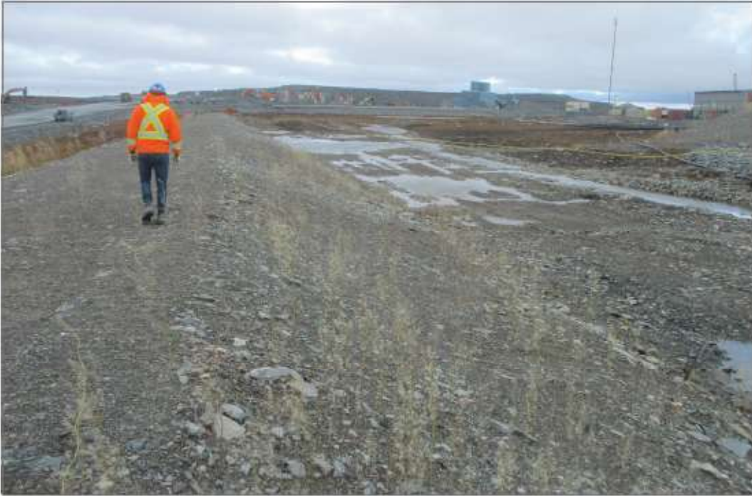
Photo 51: Berm 3—Ponded water against upstream embankment. Vegetation on Berm.
