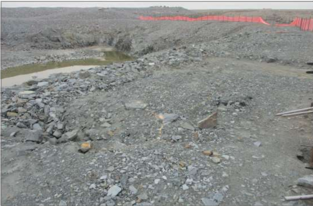
Photo 10: Pond CP3 - Looking north, settlement and erosion at overburden crest.
