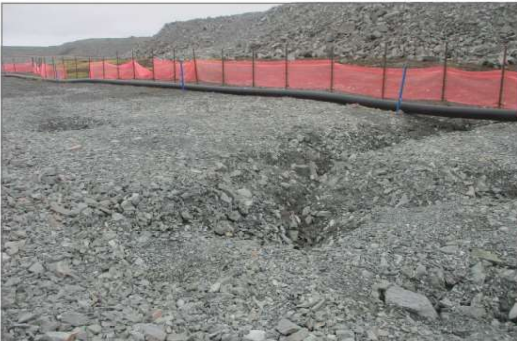
Photo 6: Pond CP4 - Northeast slope, settlement in area between rockfill covered slope on original ground.
