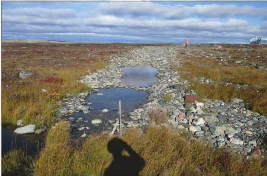
Photo 11: Channel 2—Some settlement in base of channel allowing water to pool.
