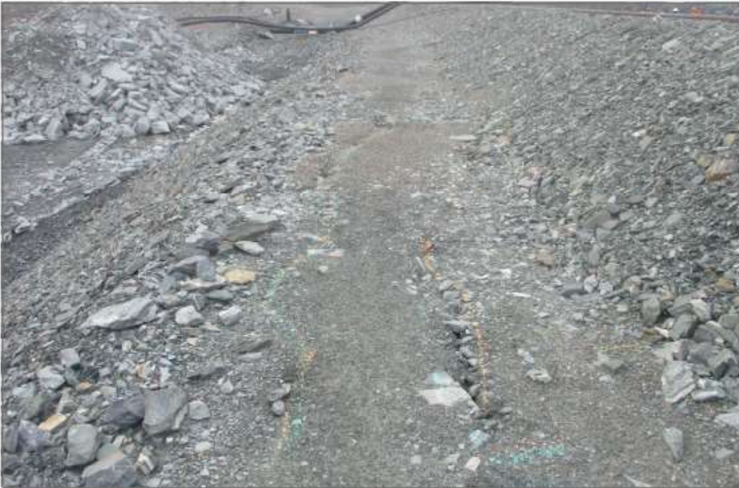
Photo 6: Dike D-CP1 - Downstream crest, minor cracking, no change from previous year.
