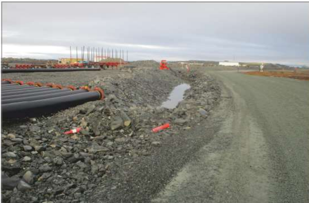
Photo 34: Culvert km 29.6 replaced with sump and pump to water storage in pit
