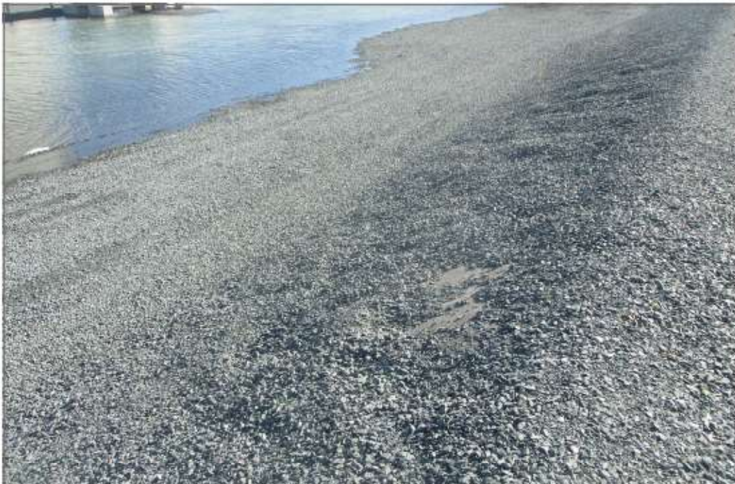
Photo 18: ITVIA Tankfarm—Exposed geotextile on south berm embankment.
