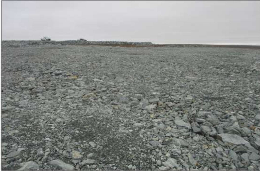
Photo 11: Berm CP4 - Undulating settlement up to 0.3 m throughout surface of berm.
