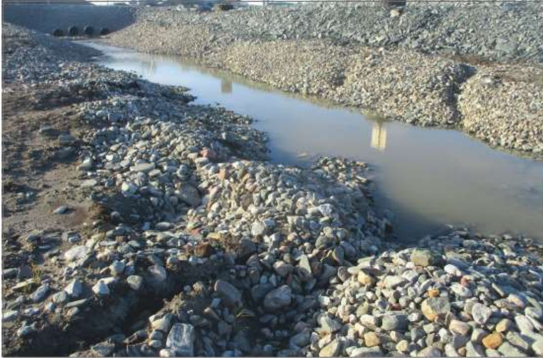
Photo 5: Channel 1—Downstream of crusher ramp, crest subsidence and erosion into channel.
