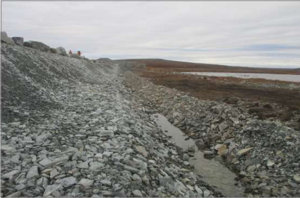
Photo 13: Dike D-CP1 - Seepage collection channel. Subsidence in base of channel.
