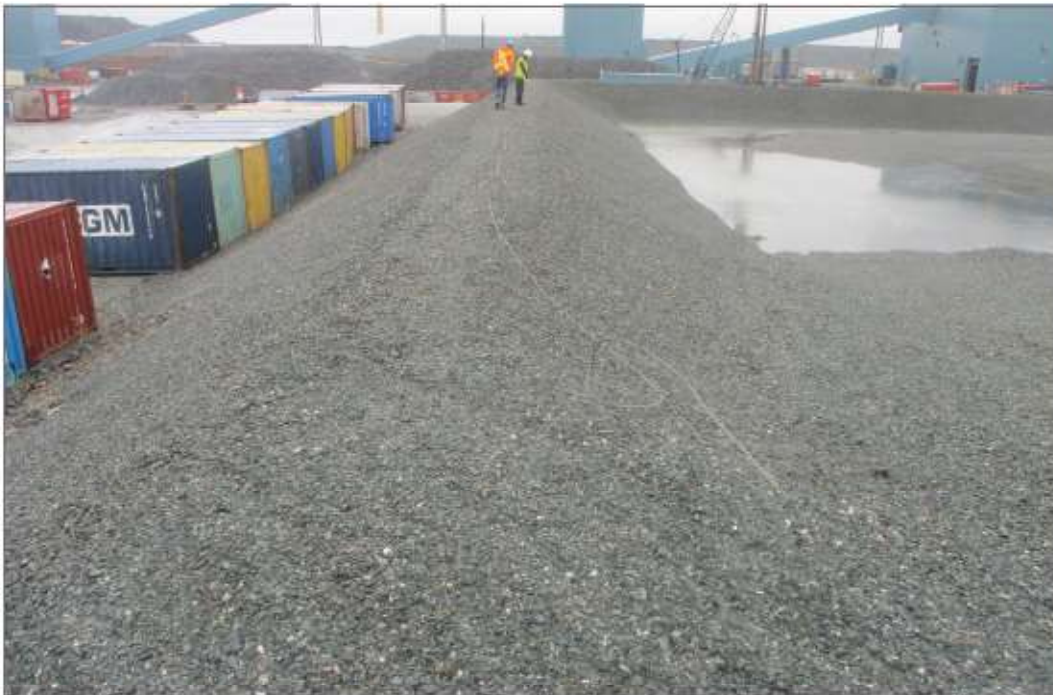
Photo 28: Industrial Fuel Storage Tanks—Exposed grounding cable on berm crest.
