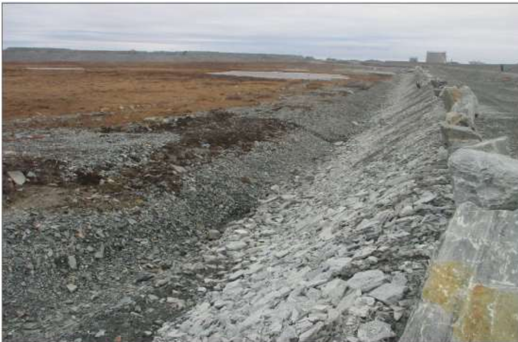
Photo 14: Dike D-CP1 - North end of disturbed ground between dike toe and seepage collection channel.
