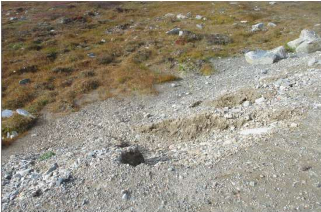
Photo 16: Emulsion Plant—west side of pad, erosion in pad slope.
