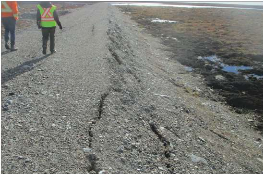
Photo 50: Berm 2—Longitudinal cracking and minor erosion along upstream embankment.
