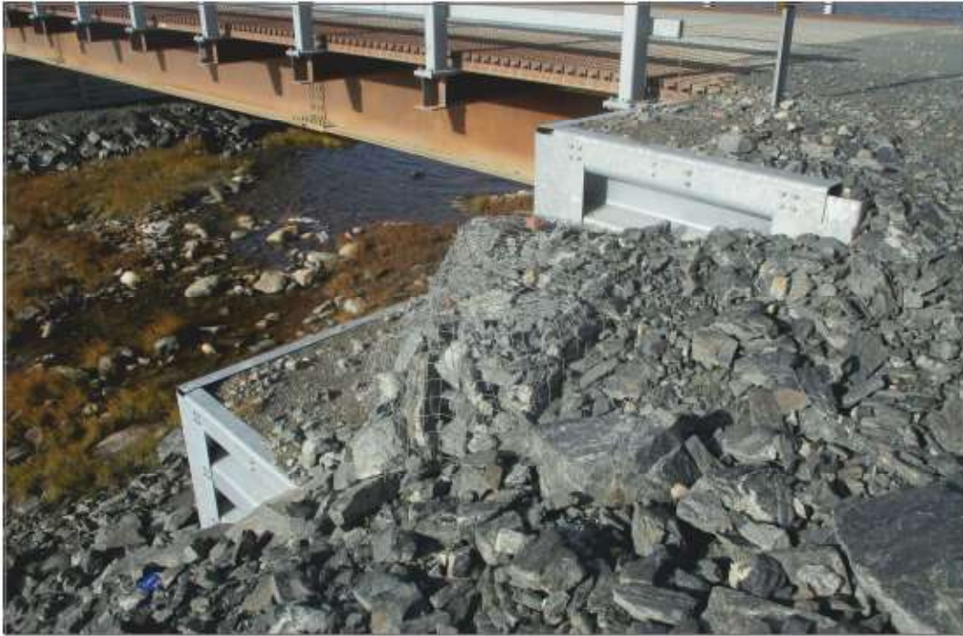
Photo 19: M-5 Bridge—Gabion North Abutment damaged
