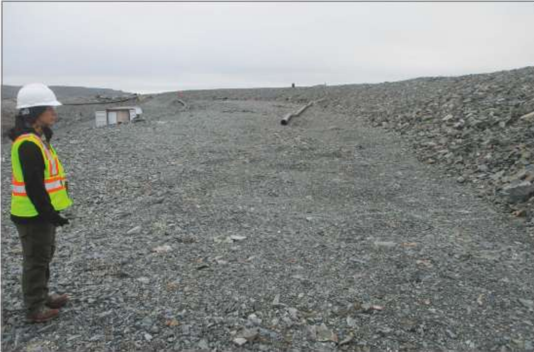
Photo 3: Pond CP3 - Looking south, rockfill covered overburden in foreground. Settlement along the overburden between CP3 and berm.
