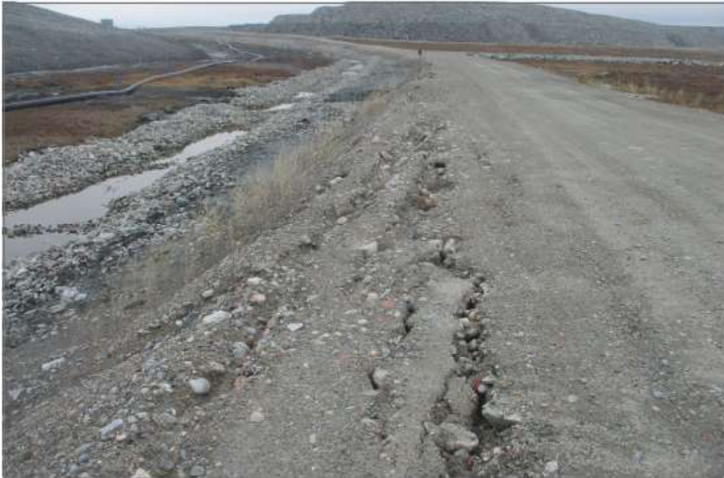
Photo 17: Channel 3—Cracking along road side slopes adjacent to channel.
