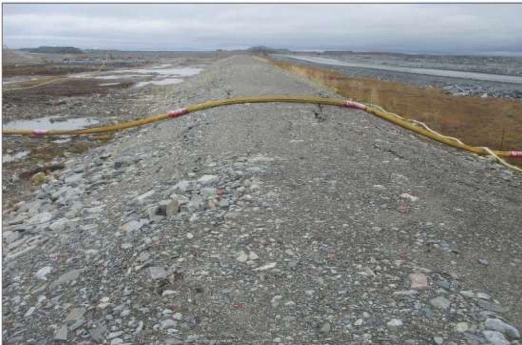
Photo 54: Berm 3—Settlement area of berm surface near west abutment.
