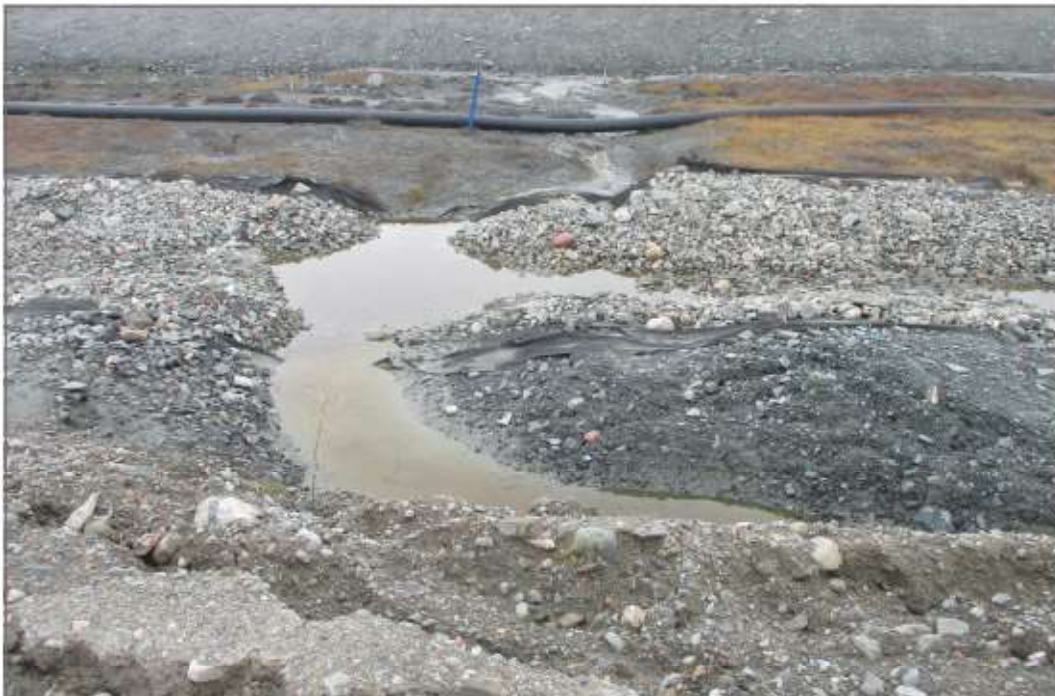
Photo 18: Channel 3—Significant subsidence across channel alignment and subsequent cracking along road side slope, looking east.
