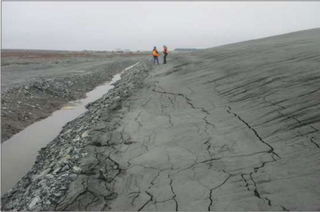
Photo 11: TSF - Sedimentation, cracking, and piping along north embankment toe.
