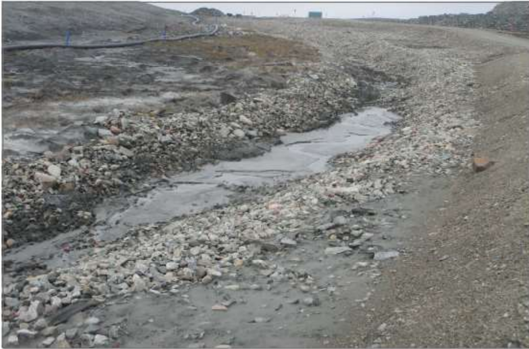
Photo 21: Channel 3—Channel base infilling with sediment, looking east.
