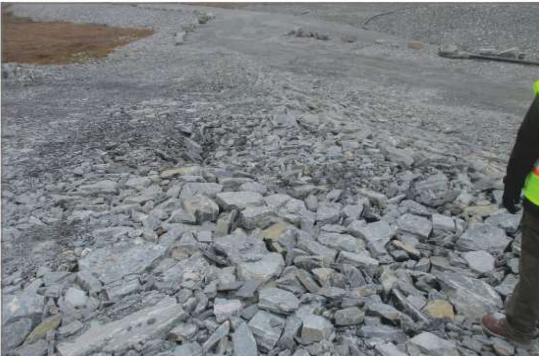
Photo 10: Pond CP2—Settlement underneath rockfill cover near ramp entry, looking south.
