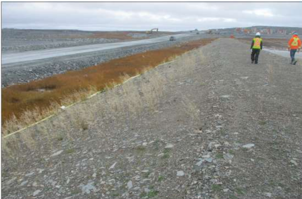
Photo 52: Berm 3—Downstream crest with vegetation growth.
