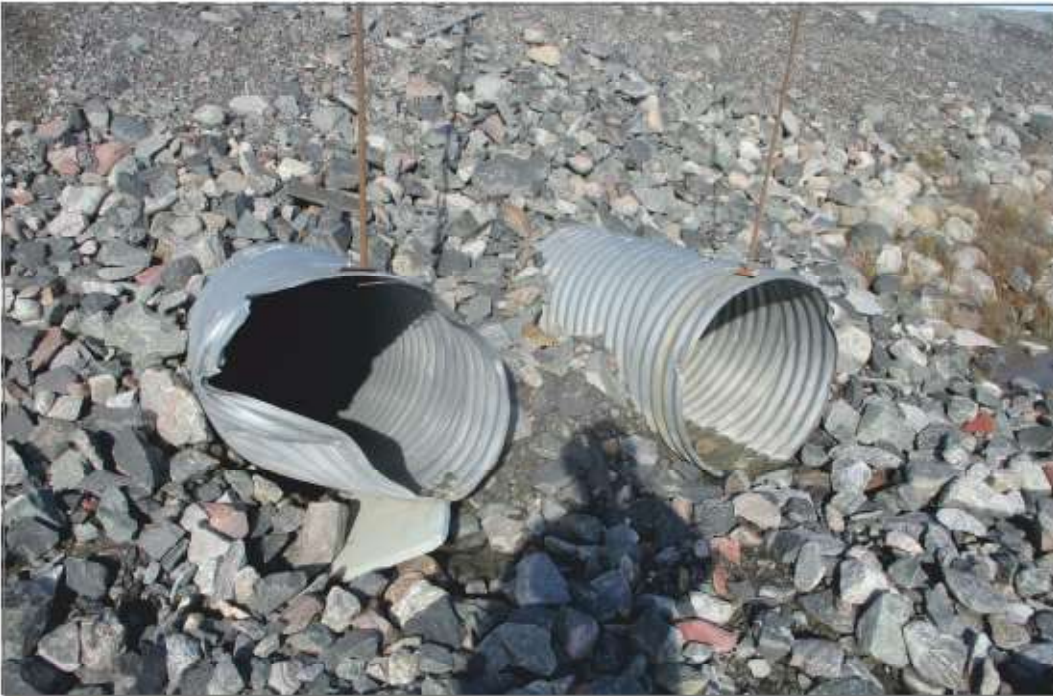
Photo 8: Culvert C13—Damage to culvert,
