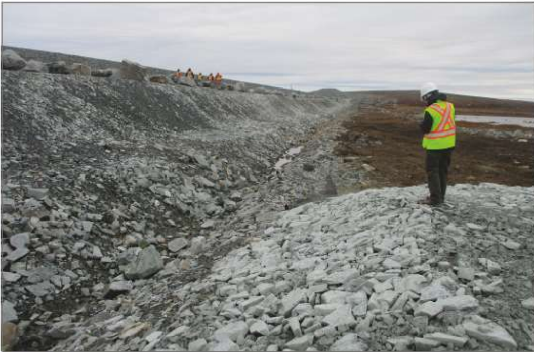
Photo 12: Dike D-CP1 - ground between the dike toe and water collection channel covered with rockfill toe berm.
