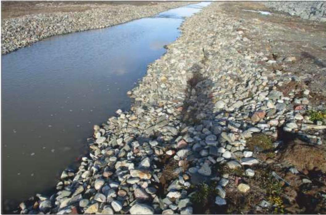
Photo 7: Channel 1—Rip settlement and cracking along crest of overburden.
