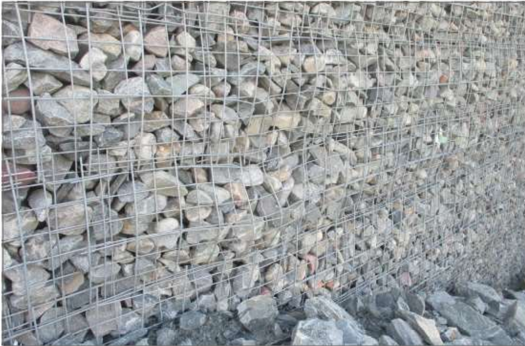
Photo 8: Crusher Pad—MSE wall, north east side. Slight localized bulge and distortion of gabion cage.
