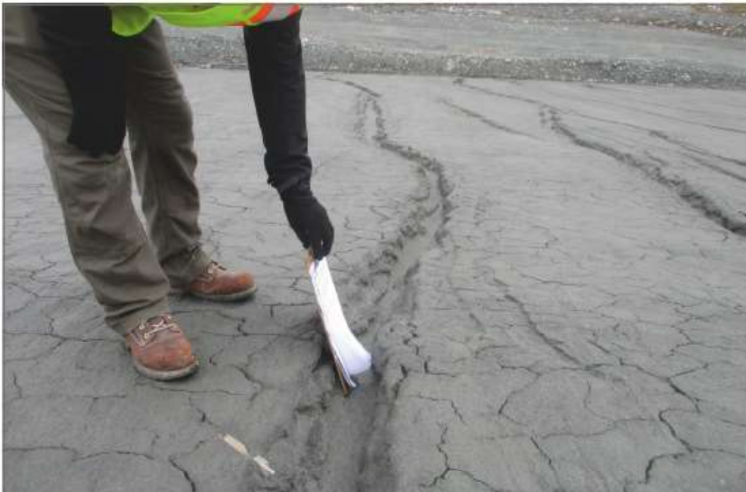
Photo 10: TSF - Erosion channels on exposed north embankment.
