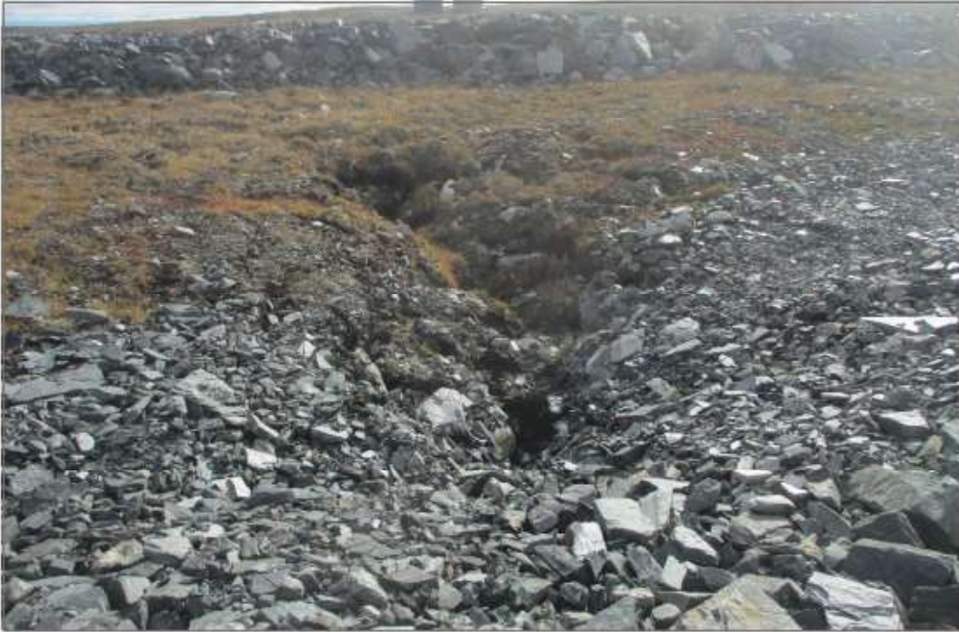
Photo 11: SP4 Saline Pond—Settlement in disturbed overburden above rockfill covered slope.
