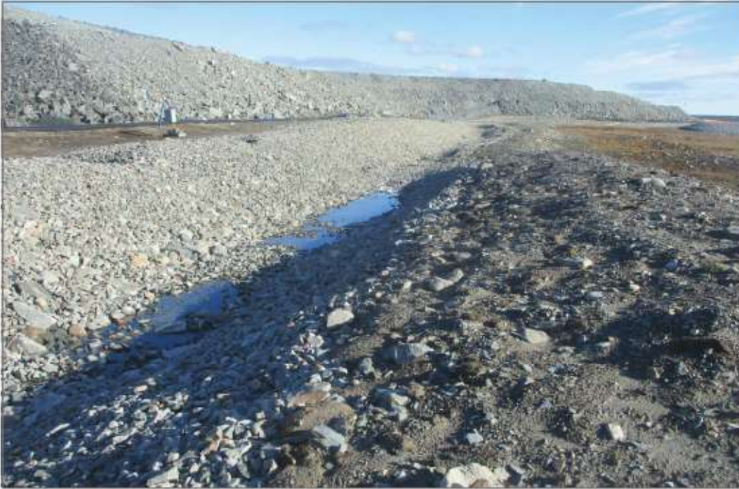
Photo 25: Channel 4 - Settlement in base of channel resulting in minor ponding.
