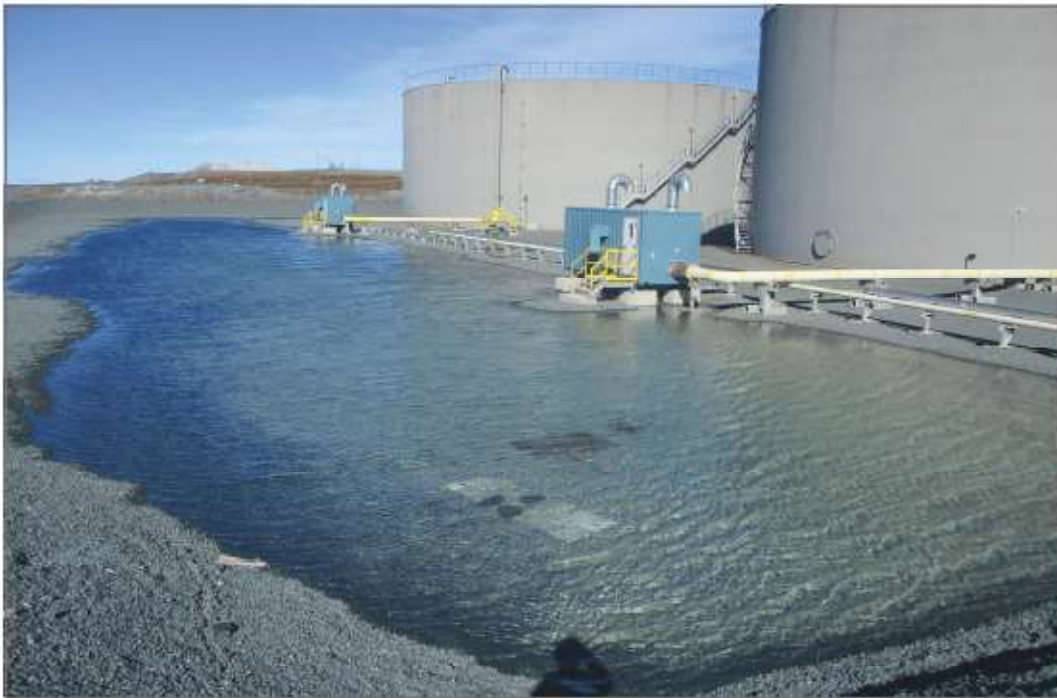
Photo 12: ITIVIA Tankfarm—Ponded water in facility.
