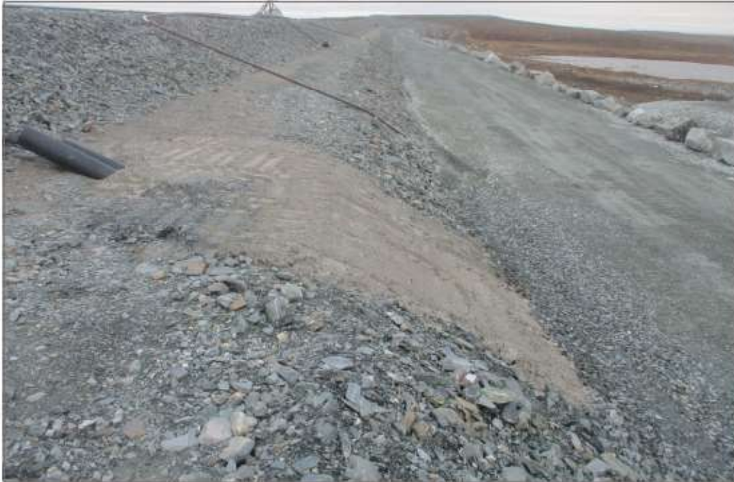
Photo 15: Dike D-CP1 - Buried line along downstream crest of dike for dewatering seepage collection pond.
