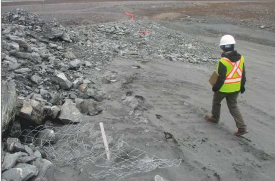
Photo 9: TSF - contact between rockfill cover and tailings at the northwest corner of Cell 1.
