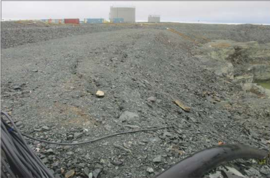
Photo 3: SP1 Saline Pond - Deformation and cracking in top of overburden protected slope, southwest corner of pond.
