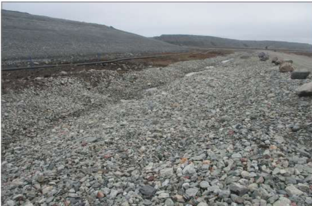
Photo 16: Channel 3—Undulating settlement along base of channel causing ponding.
