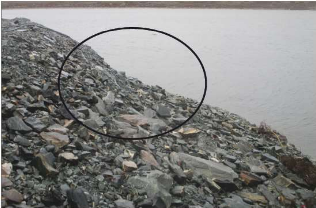
Photo 18: Dike D-CP1 Jetty 1—Erosion at southeast corner—under cutting top portion of fill. No change from previous years.
