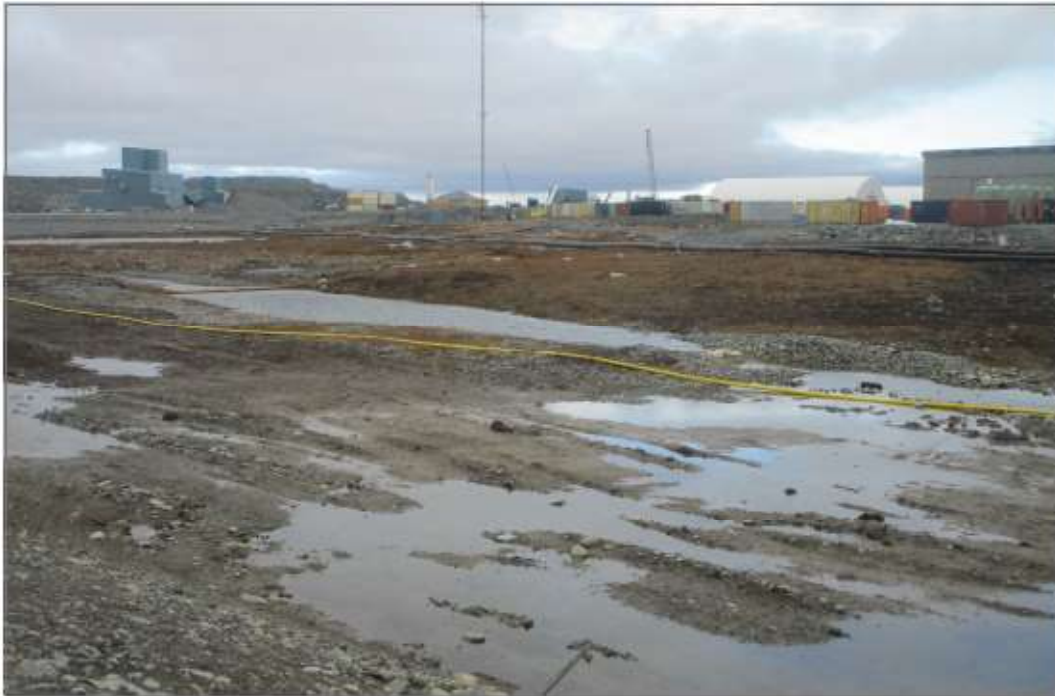
Photo 31: Channel 5—Upper reach, south of Portal2, significant subsidence and cracking along slopes with rip rap settled below water level in channel.
