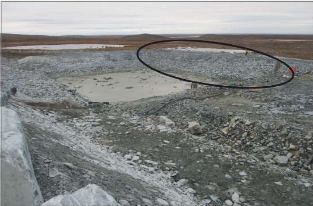
Photo 10: Dike D-CP1 - Seepage collection pond downstream of dike. Deformation of fill at southeast corner of pond has been rebuilt and rockfill cover placed on exposed tundra.
