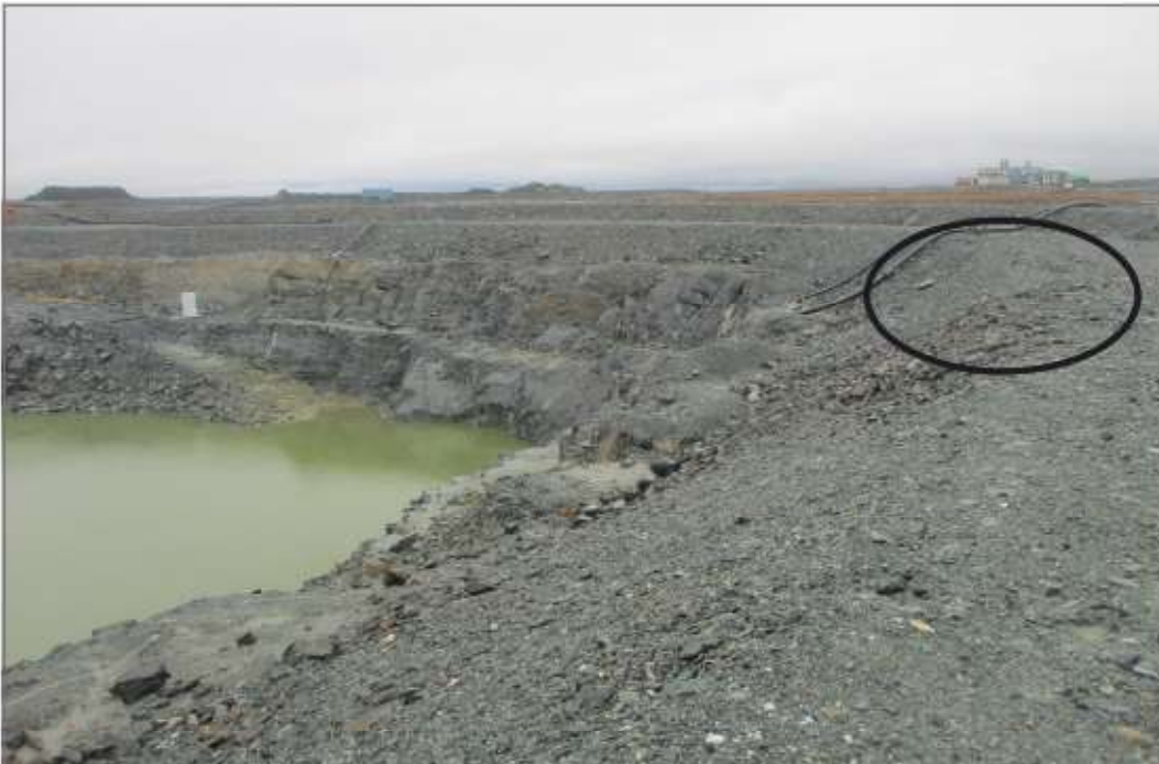
Photo 4: SP1 Saline Pond - Overview of deformation and cracking in top of overburden protected slope, southwest corner of pond.
