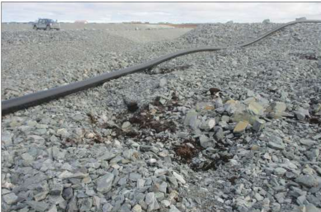
Photo 42: Channel 9—Thermal subsidence between rip rap and original ground interface.
