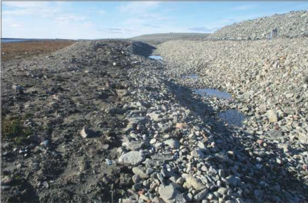
Photo 27: Channel 4 - Subsidence in downstream slope (west slope) of channel.
