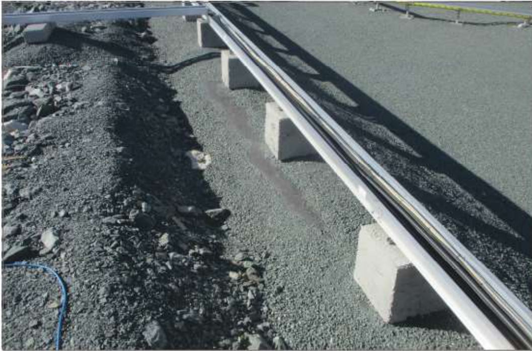
Photo 13: ITIVIA Tankfarm— Geotextile exposed along south berm crest.
