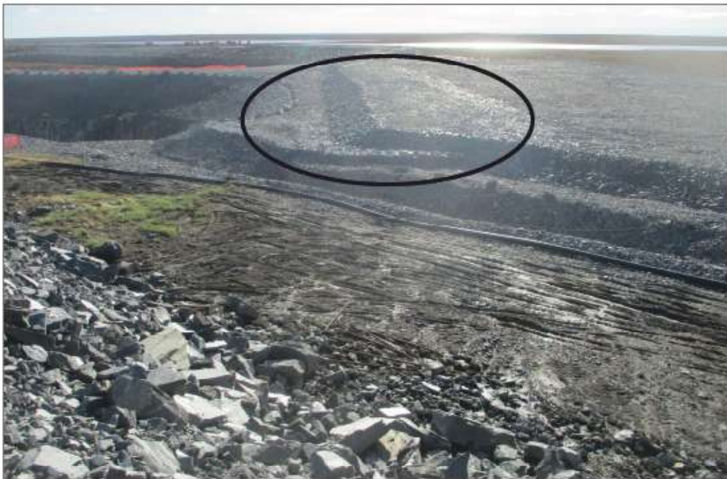
Photo 8: Pond CP4 - North slope, Rockfill placed in area between rockfill covered slope and thermal berm in 2022.
