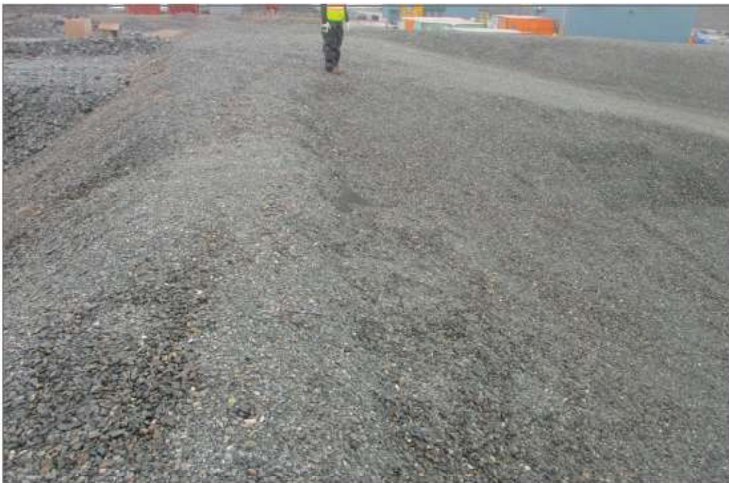
Photo 30: Industrial Fuel Storage Tanks—Exposed geotextile along inside of berm.
