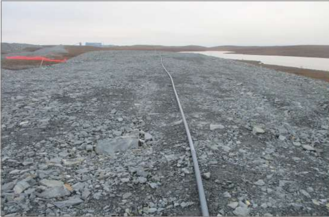
Photo 7: Berm CP2—Surface of berm looking north. GTC instrumentation installed on berm.
