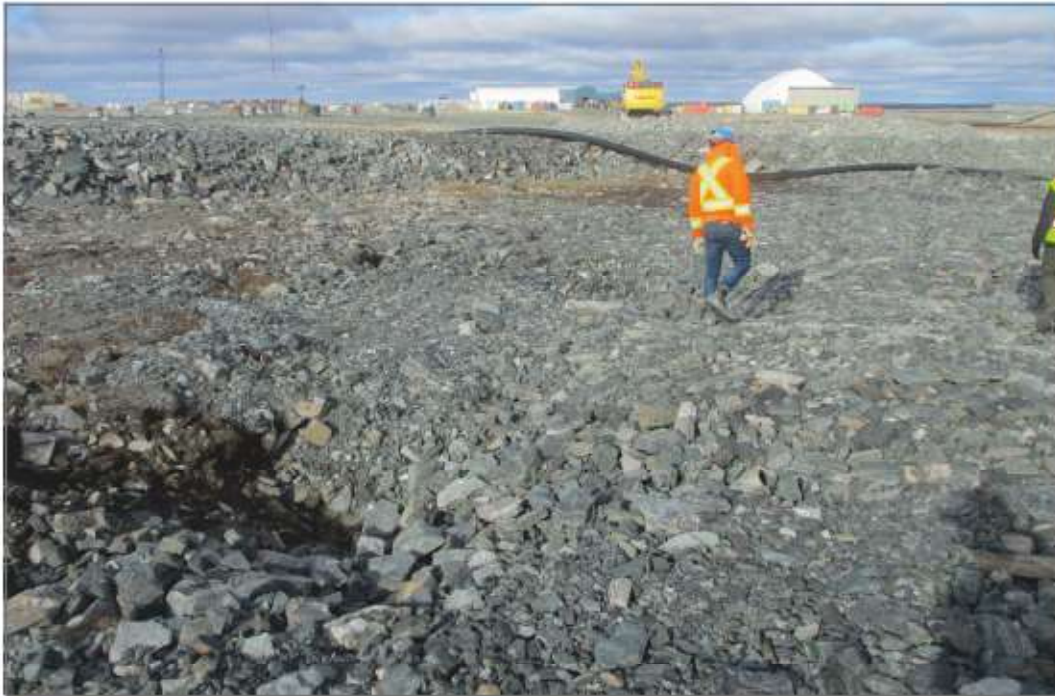
Photo 14: SP4 Saline Pond—Thaw subsidence underneath rockfill covered overburden slope.
