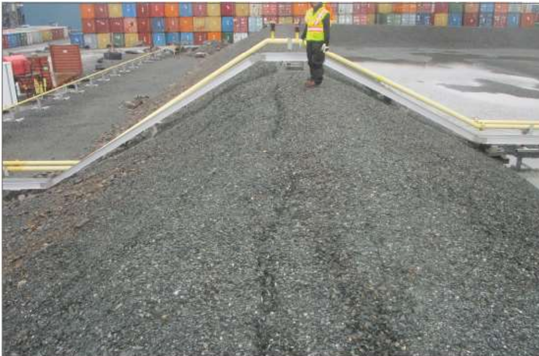
Photo 26: Industrial Fuel Storage Tanks—Cracking on top of berm. Settlement and erosion under pipe infrastructure.
