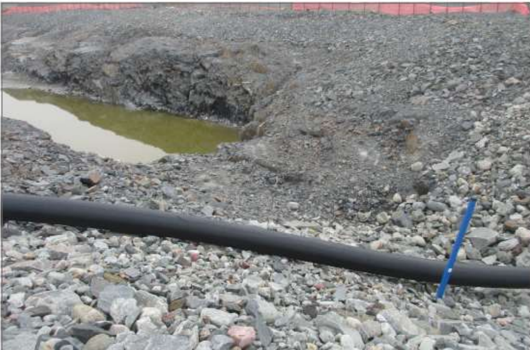
Photo 14: Channel 3—Discharge into CP3.
