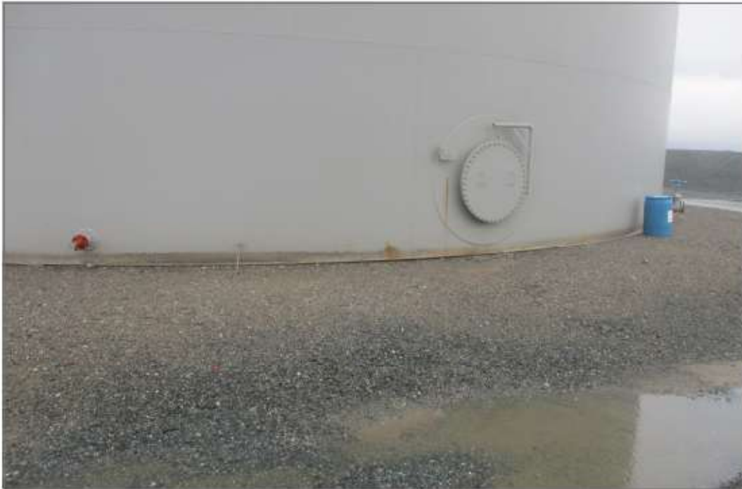
Photo 29: Industrial Fuel Storage Tanks—Small amount of erosion on tank pedestals.
