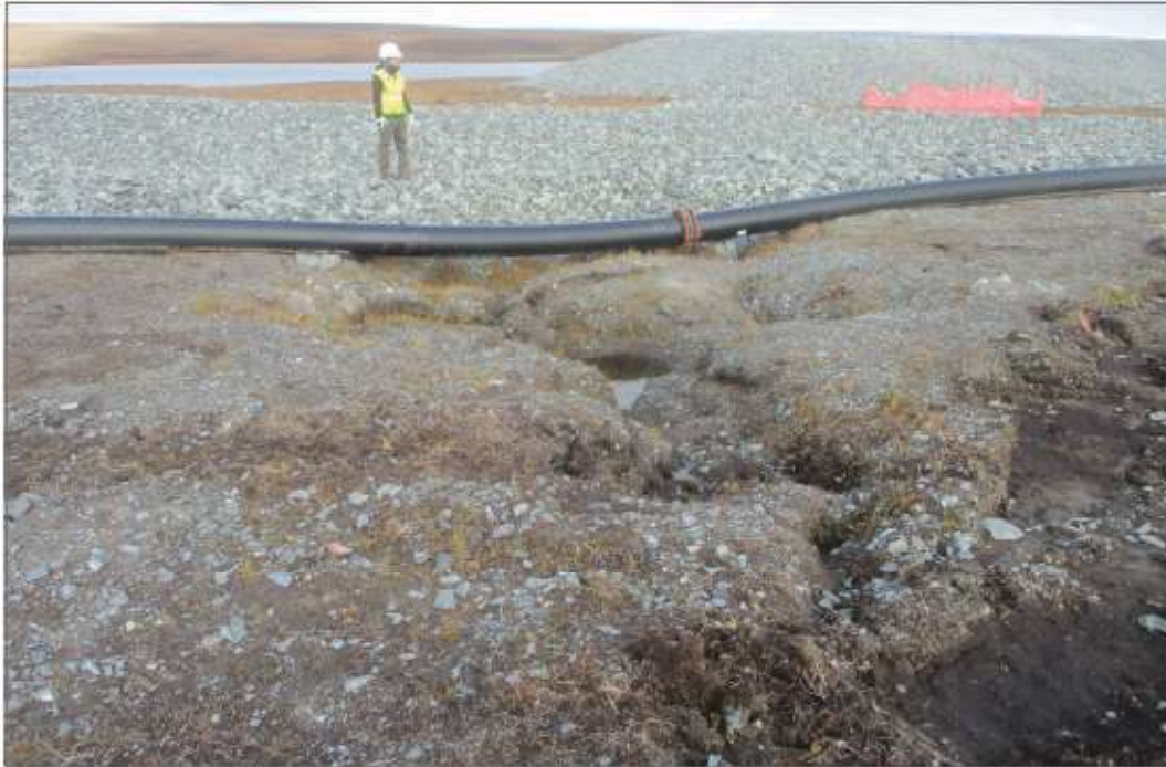
Photo 41: Channel 9—Thermal degradation of original ground upstream of channel.
