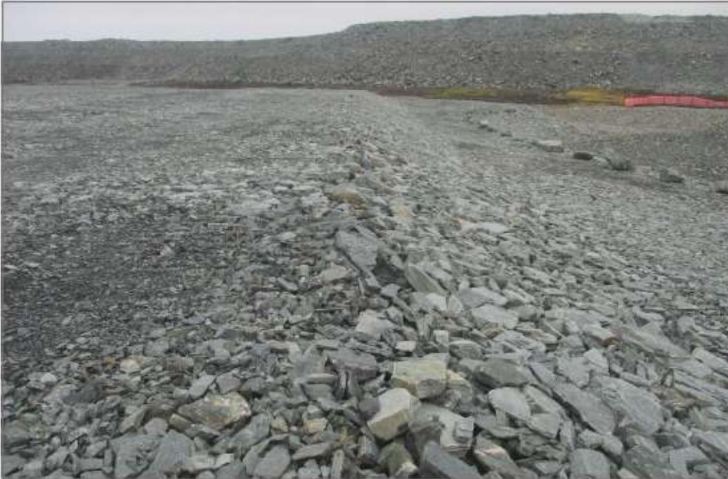
Photo 9: Pond CP4 - Rockfill placed between CP4 slope and berm to reduce thaw subsidence observed in 2021 inspection.
