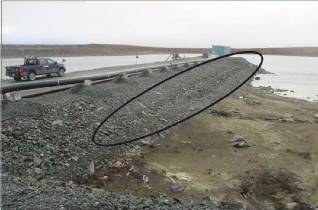
Photo 17: Dike D-CP1 Jetty 1 - Erosion at south east side of Jetty 1. No change from previous years.
