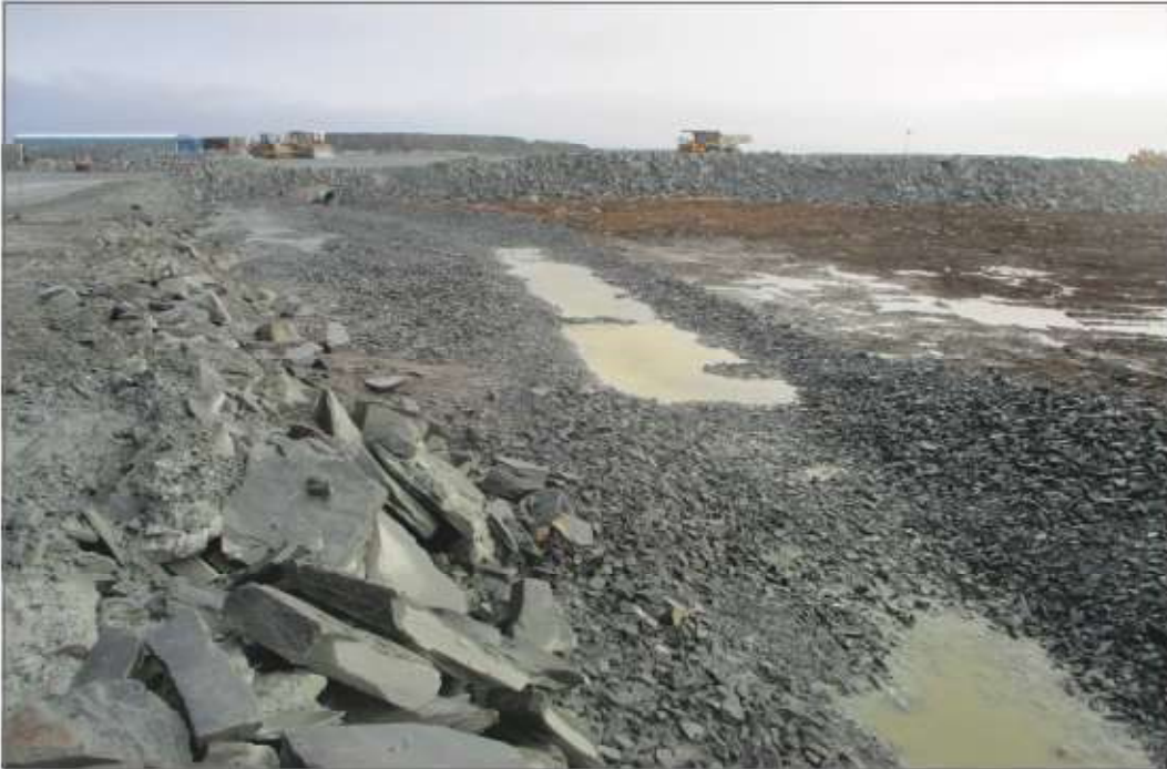
Photo 35: Channel 7—Upper reach, minor subsidence and pooling at bottom of channel, looking north.
