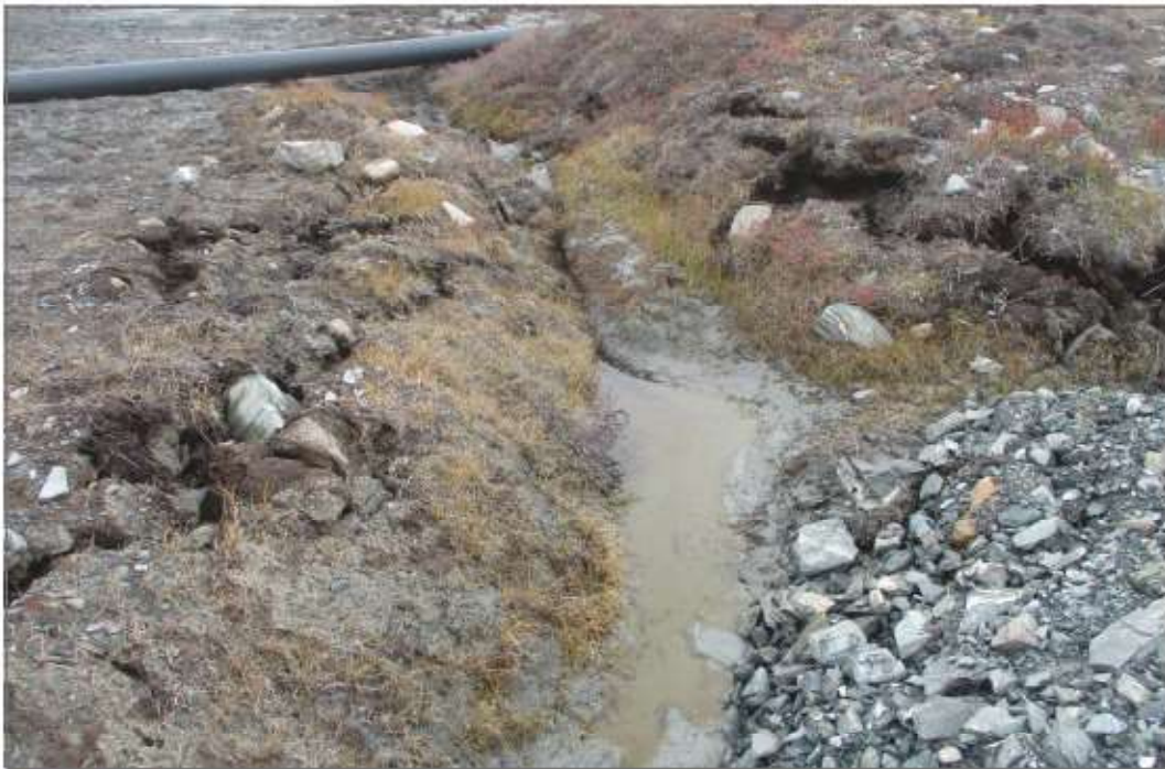
Photo 20: Channel 3—Thermal degradation of ground upstream of Channel 3.
