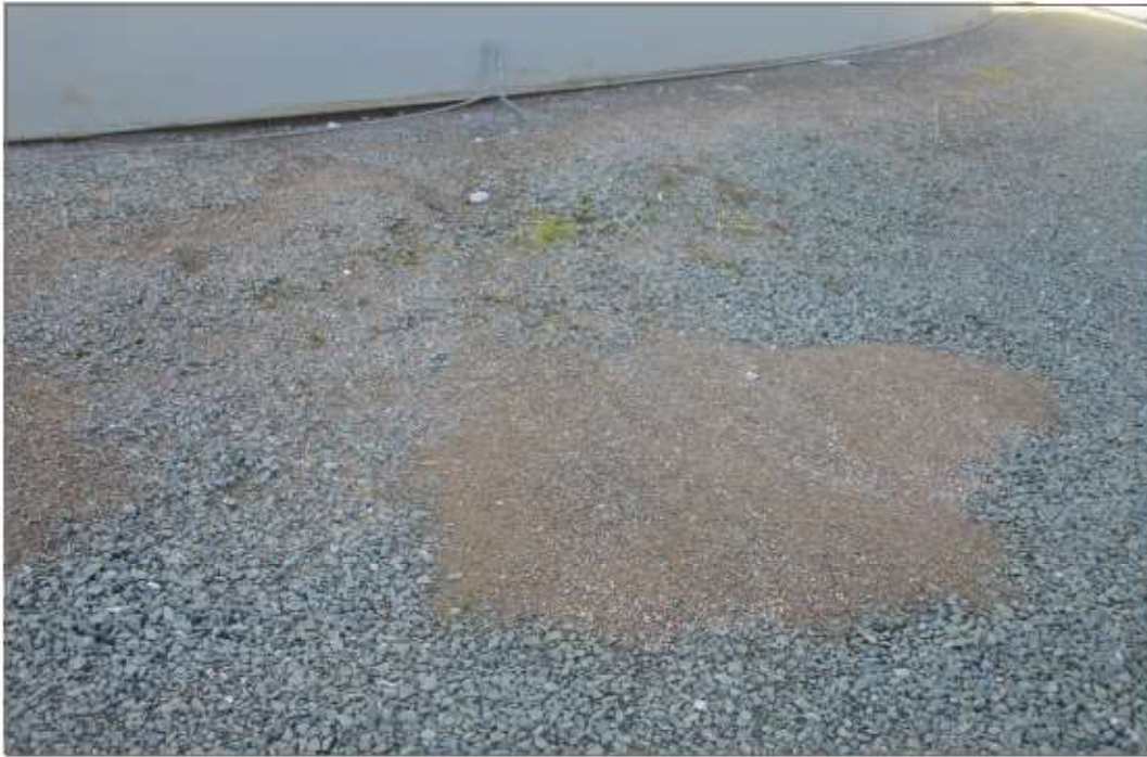
Photo 15: ITIVIA Tankfarm—Fines erosion on edge of tank pedestal.
