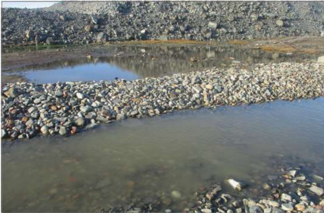
Photo 8: Channel 1—Standing water adjacent to channel slope and ore pad.
