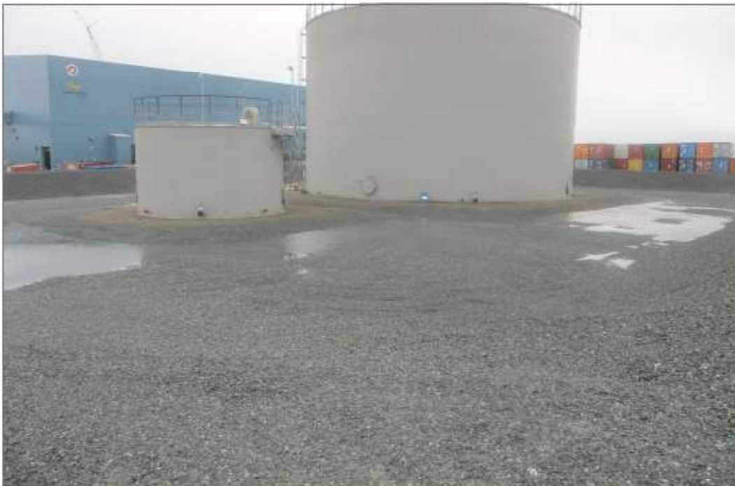
Photo 24: Industrial Fuel Storage Tanks.
