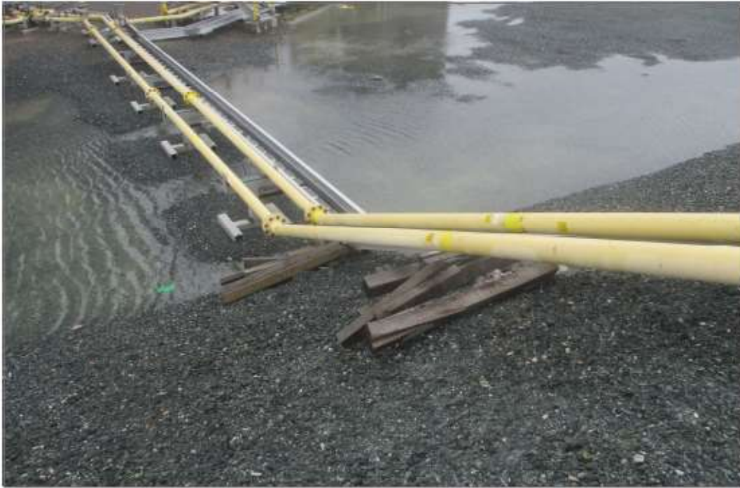
Photo 27: Industrial Fuel Storage Tanks—Collapsed pipe support on berm crest.
