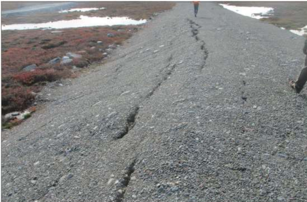
Photo 48: Berm 2—Longitudinal cracking along downstream slope and crest .
