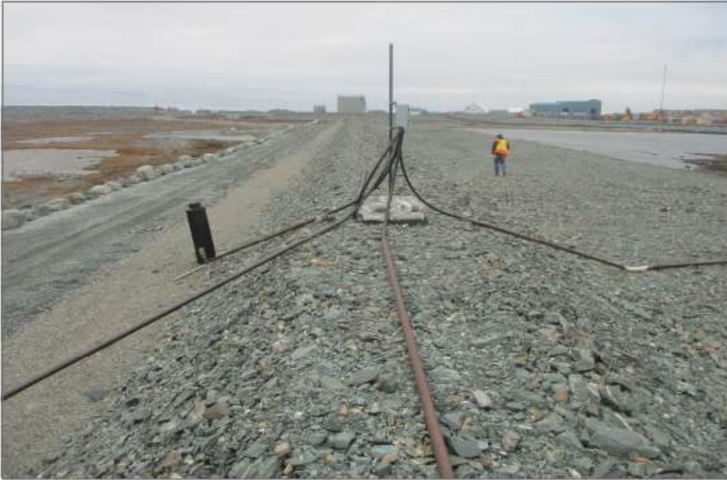
Photo 5: Dike D-CP1 - Crest—Center and downstream. GTC housing and datalogger.
