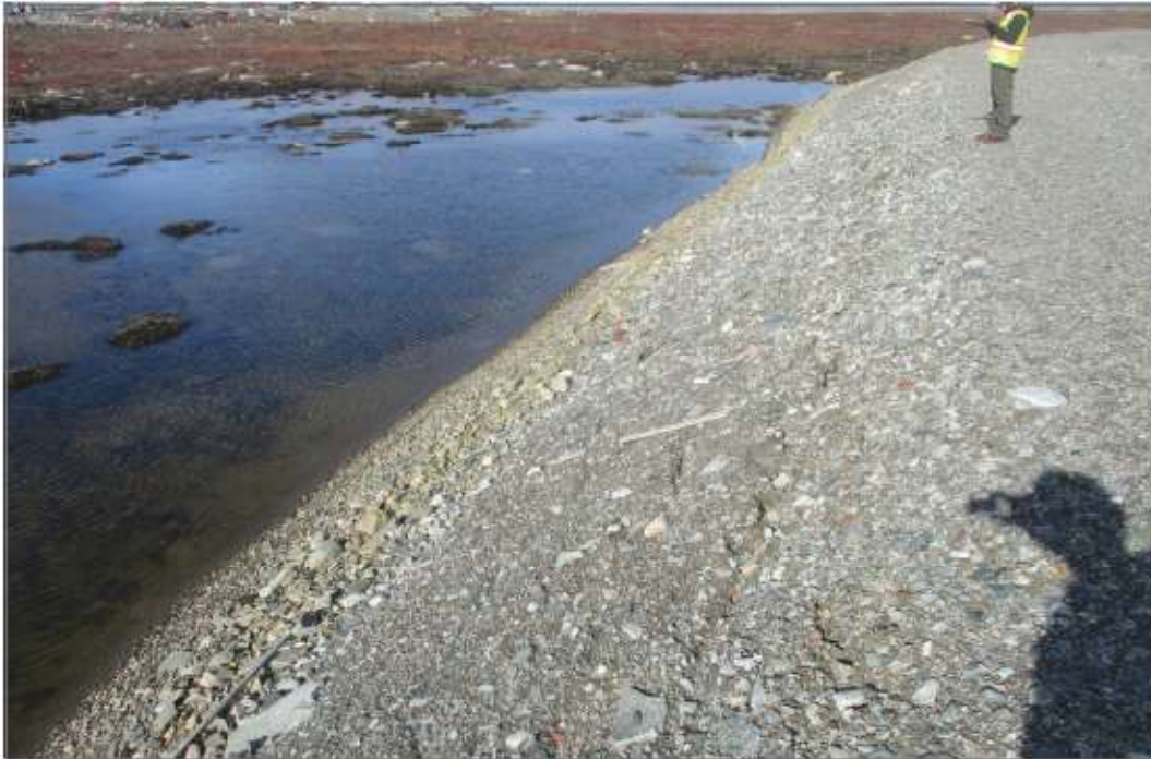
Photo 49: Berm 2—Impounded water against upstream side of Berm 2 with high water mark.
