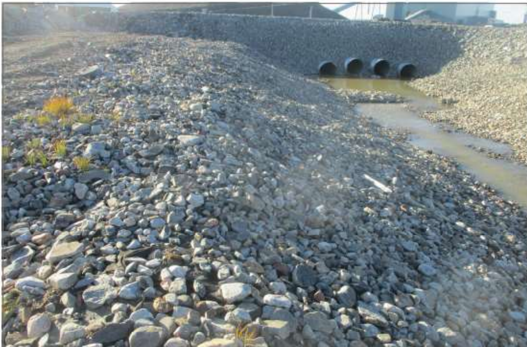
Photo 4: Channel 1—Downstream of crusher ramp, crest subsidence and erosion into channel.
