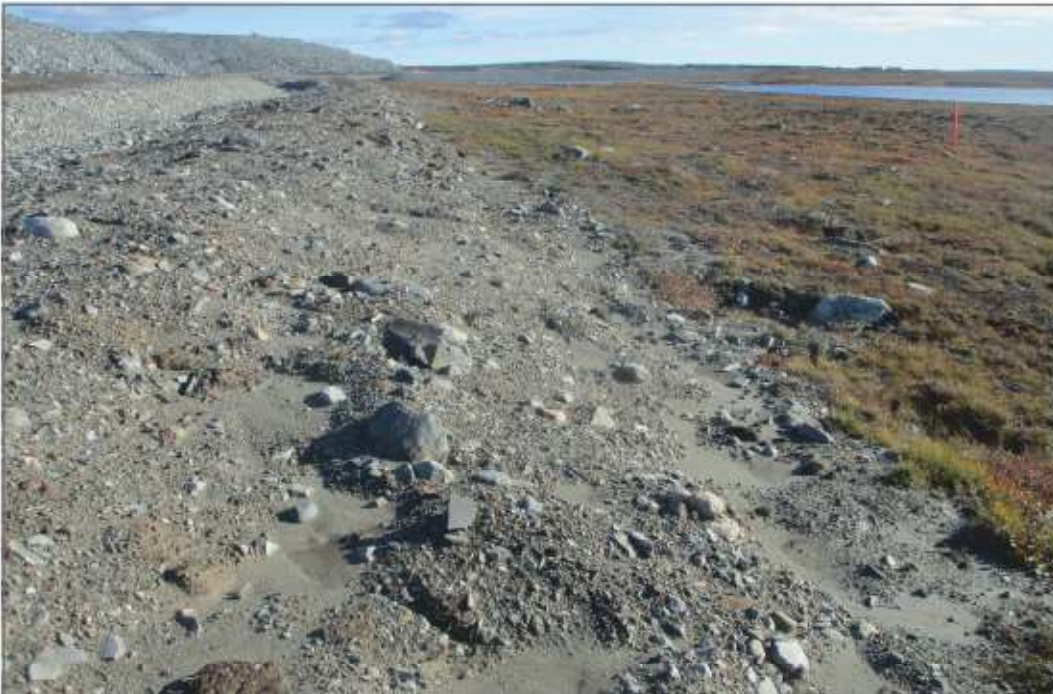
Photo 28: Channel 4 - Migration of fines from un-armoured overburden berm.
