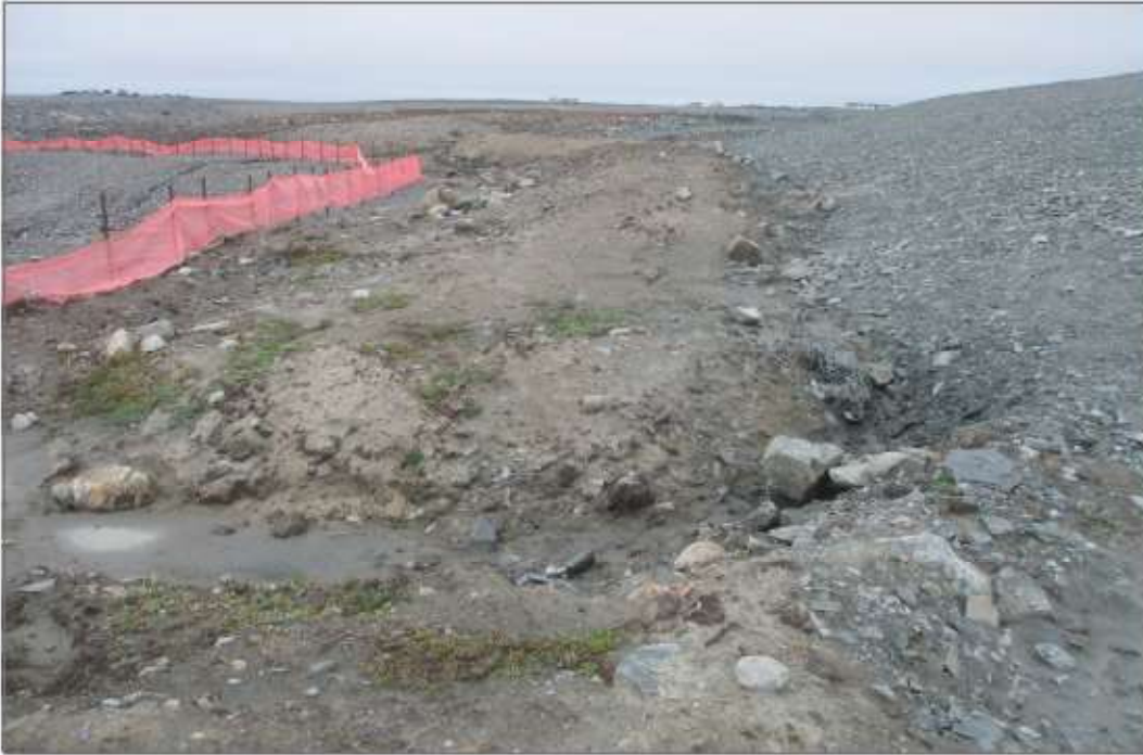
Photo 5: Pond CP3 - Runoff/erosion channels into pond from north end of TSF drainage, located on north side of pond.
