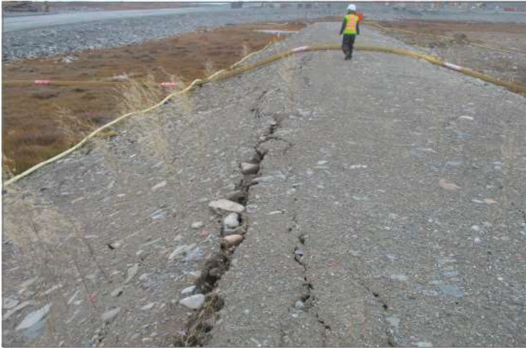
Photo 53: Berm 3—Cracking along slopes and crest.
