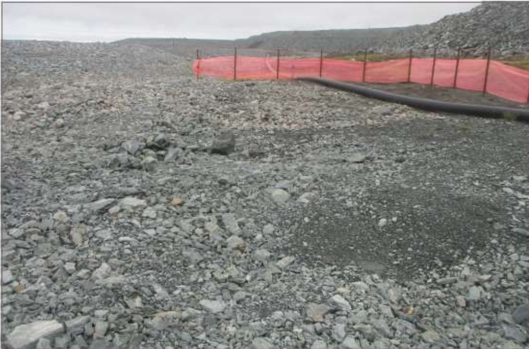
Photo 5: Pond CP4 - Settlement and cracking above east slope.
