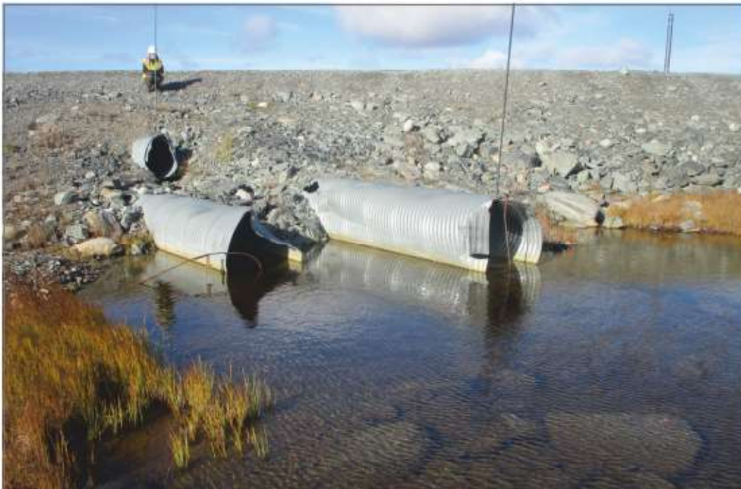
Photo 8: Culvert km 7.4—Damage to culvert inlets
