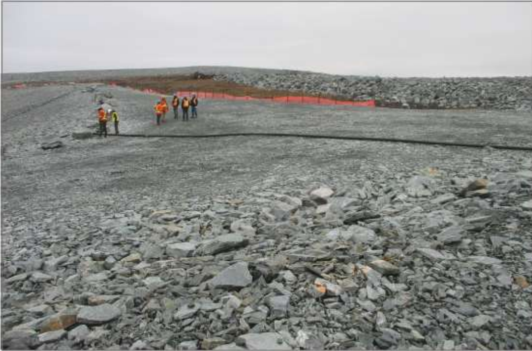
Photo 13: Pond CP4 - Rockfill cover placed over native ground above slopes of CP4.
