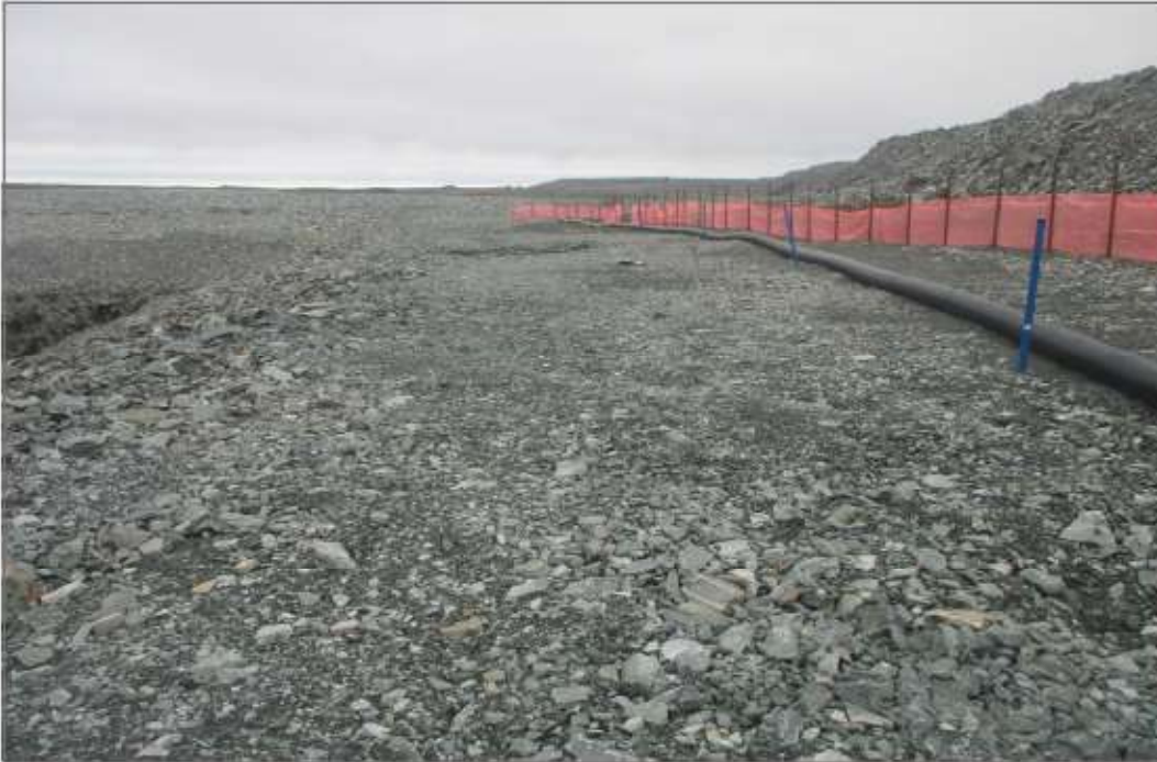
Photo 7: Pond CP4 - Ground above rockfill covered overburden slope. Settlement and subsidence in the area.
