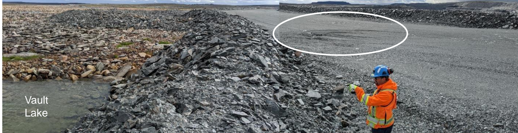
Area 2 Looking South with Subsidence Circled
