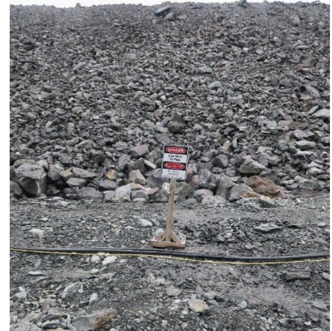
Seepage from Toe of Dump
