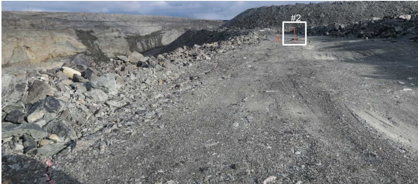
Tension Cracks at Crest by Extensometer #2, Looking North
