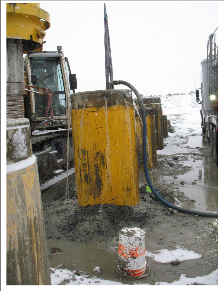
Photo No. 5 Overflow of water during tremie filling of secant piles with Cement-Bentonite slurry
