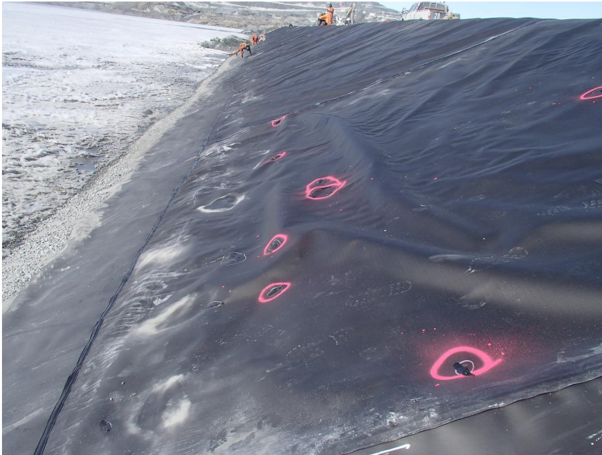
Photograph CD-1879: From Sta. 0+735/-28 m, looking N. View of the repaired holes on panel 850.
