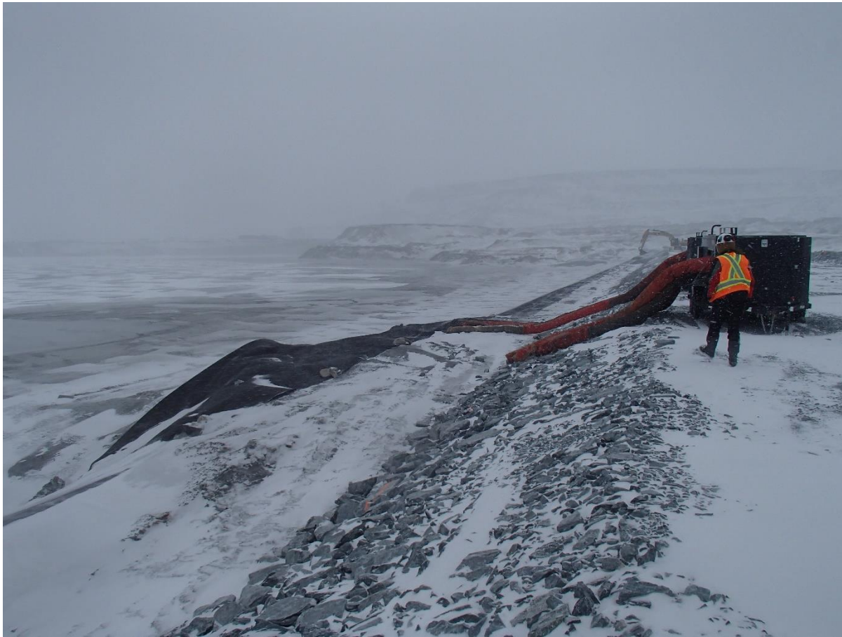
Photograph CD-1828: From Sta 0+410/-22 m, looking N. Defrosting of the deposition finger materials with two Frost Fighters at Sta. 0+390 m.
