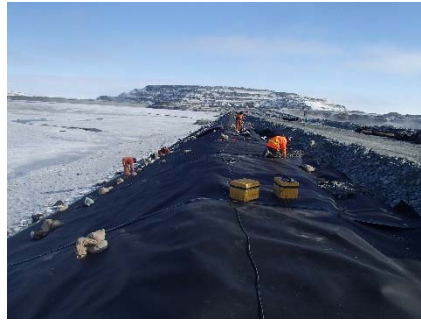
CD-1872 (2018-05-28), looking N from Sta. 0+900/-24 m. Installation of the LLDPE liner on the upstream slope 2H:1V between El. 143 m and 145 m from Sta. 0+900 m to 0+760 m (panel numbers 824 to 844).
