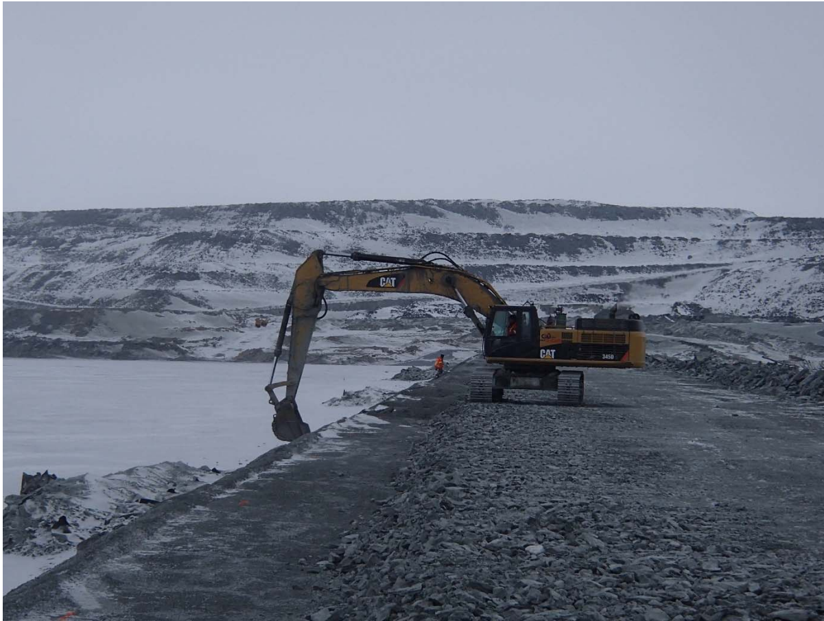
Photograph CD-1846: From Sta. 0+835/-25 m, looking N. Profiling of the upstream slope (2H:1V) from El. 143 to 145 m with an excavator between Sta. 0+330 and 0+600 m and between Sta. 0+715 m and 40+730 m. The removed material was placed with material from the fine filter stockpile on the fourth 0.5 m thick lift of fine filter from El. 144.5 m to 145 m upstream of the coarse filter with an excavator from Sta. 0+330 m to 0+600 m and between Sta. 0+715 m and 40+730 m.
