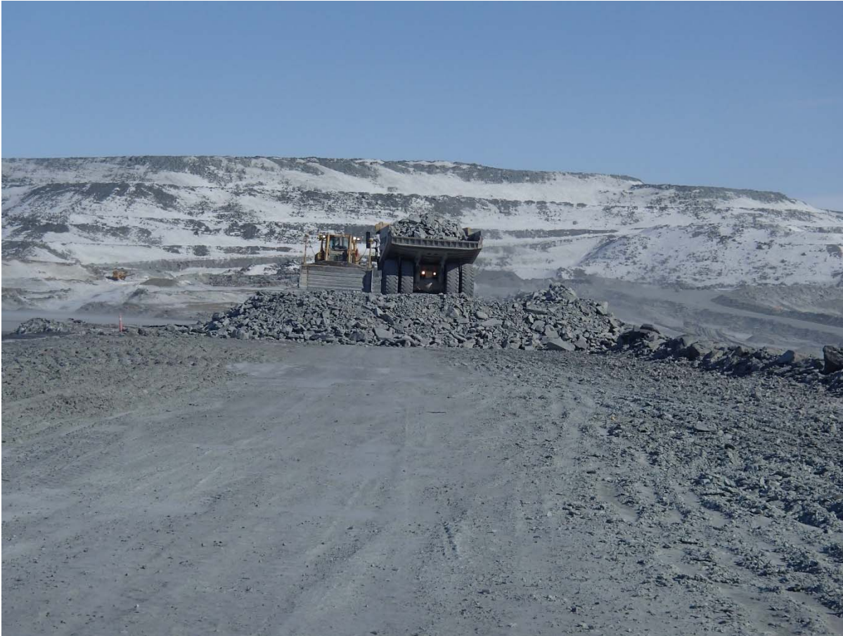
Photograph CD-1802: From Sta. 0+770/-16 m looking N. Placement a 2 m thick (approx.) lift of intermediate volcanic (IV) rockfill from El. 143 m to El. 145 m from approx. Sta. 0+525 to 0+710 m (o.s. -28 to -18 m).
