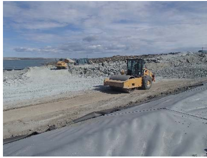
SD3-351 (2018-07-18), looking SE from Sta. 20+740/-24 m. Compaction of the layer of compacted sieved till placed against the upstream slope from Sta. 20+599 m to 20+613 m.
