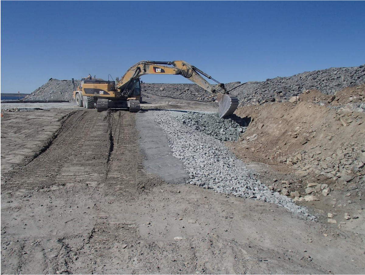
Photograph SD3-341: From Sta. 20+600/-58 m, looking W. Placement of a first 0.5 m thick lift of fine rockfill on the upstream slope of the upstream toe liner tie-in with an excavator from Sta. 20+588 m to 20+599 m.
