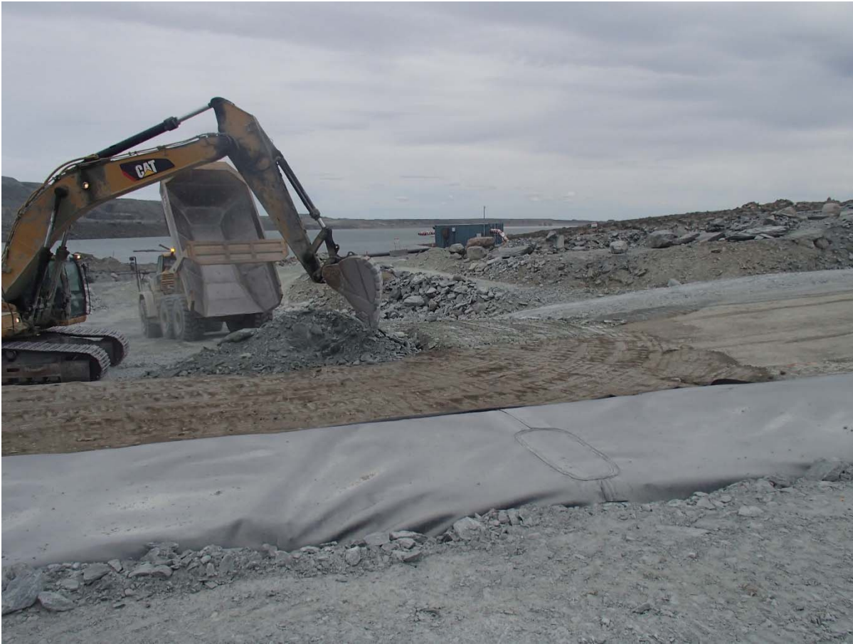
Photograph SD3-346: From Sta. 20+760/-21 m, looking E. Placement of a third 0.5 m thick lift of fine UM rockfill (0-500 mm) upstream of the low quality till (0-150mm) from El. 143 m to 143.5 m from Sta. 20+668 m to 20+777 m.
