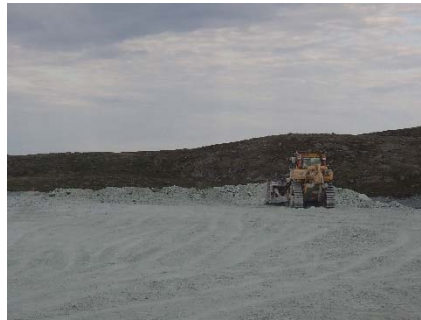
NCIS-122 (2018-07-27), looking W from Sta. 1+960/-6 m (approx.). Placement of a 2 m thick (approx.) lift of UM rockfill from El. 152 m to El. 154 m (approx.) with a dozer from Sta. 1+830 m to 1+860 m (+8 m to -23 m).
