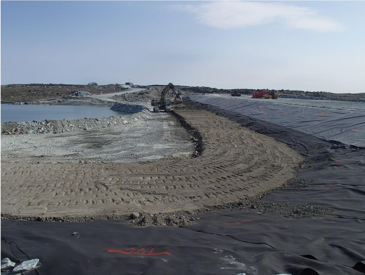
Photograph SD3-323: From Sta. 20+610/-43m, looking S. Placement of the first lift of low quality till (0-150 mm) from El. 142 m to 142.5 m from Sta. 20+610 m to 20+715 m.
