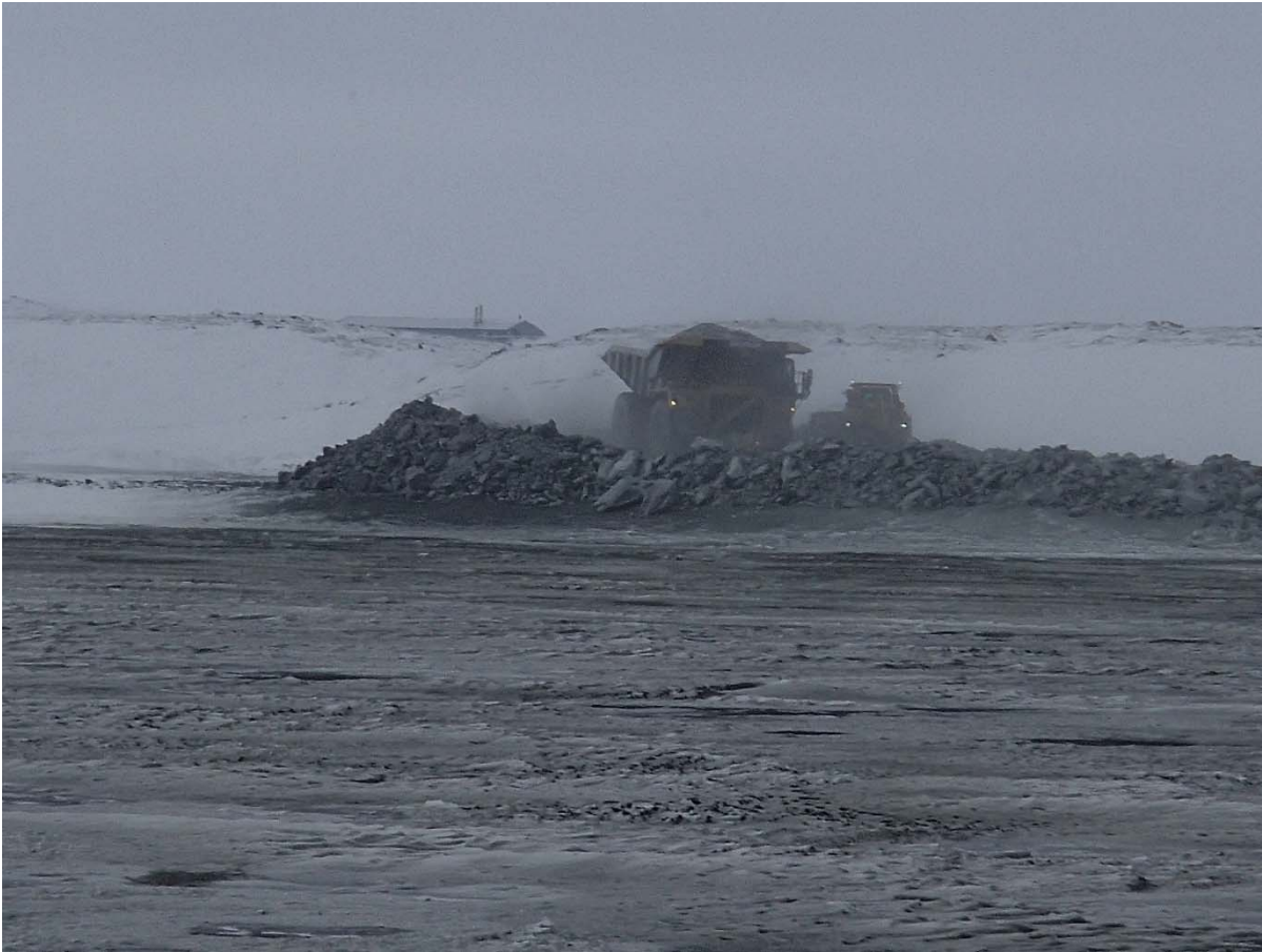
Photograph NCIS-008: Placement a 2 m thick (approx.) lift of UM rockfill from El. 150 m to El. 152 m (approx.) with a dozer. The material is of good quality and is well graded.
