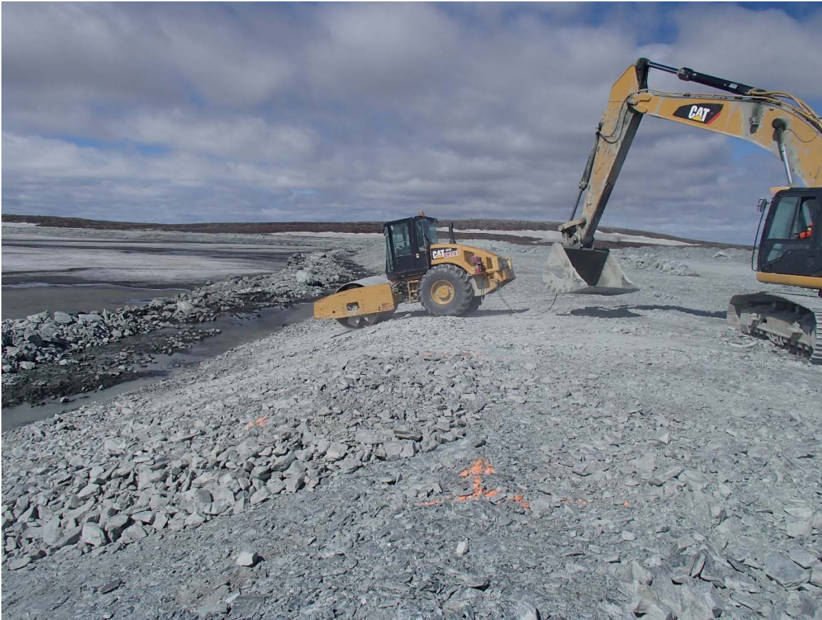
Photograph NCIS-035: From Sta. 2+550/-25 m (approx.), looking N. Compaction of the 0.5 m lift (approx.) of coarse filter between El. 150 and 152 m with a 10-tonne smooth-drum compactor (4 passes) in the upstream slope from Sta. 2+524 m to 2+450 m.
