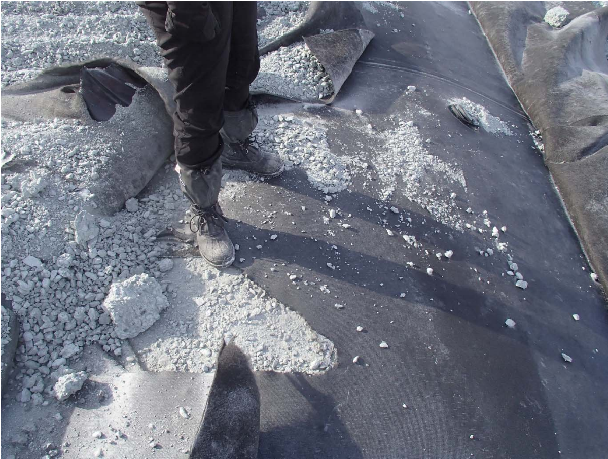
Photograph CD-1833: From Sta. 0+390/-25 m, looking S. Damaged geomembrane near a deposition finger on Central Dike at Sta. 0+390 m.
