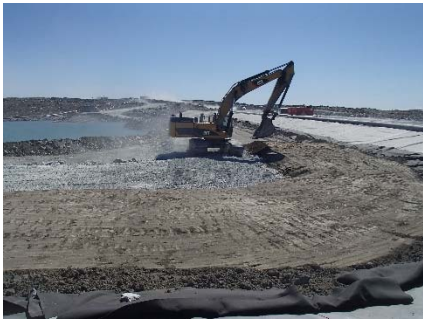
SD3-344 (2018-07-16), looking S from Sta. 20+610/-43 m. Placement of a third 0.5 m thick lift of low quality till (0-150 mm) from El. 142.5 m to 143 m from Sta. 20+570 m to 20+590 m.
