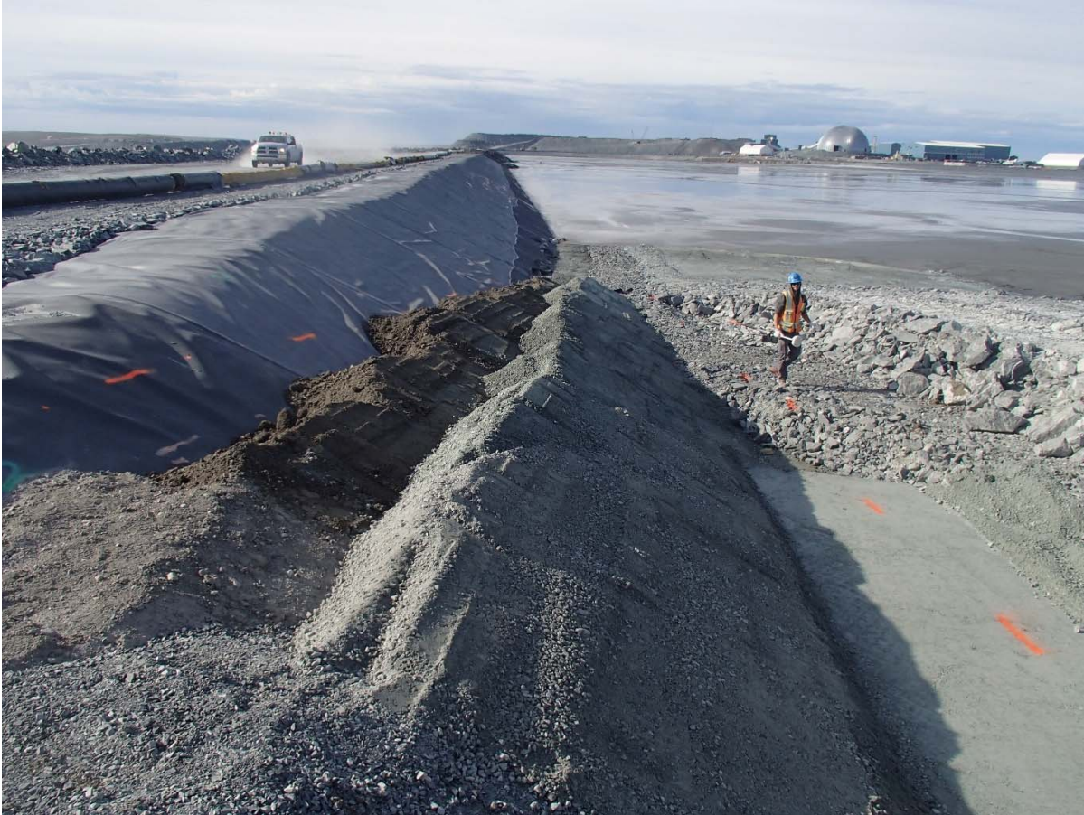
Photograph CD-1896: From Sta. 0+140/-30 m, looking S. Placement of 0.5 m thick layers of compacted sieved till and fine filter on the upstream slope of Central Dike with an excavator from Sta. 0+147 m to 0+177 m.
