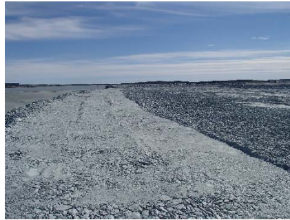
NCIS-050 (2018-06-26), looking S from Sta. 1+230/-55 m. Compaction of the 1.5 to 2 m lift (approx.) of ultramafic (UM) rockfill at El. 150 m with a 10-tonne smooth-drum compactor with vibration (6 passes) between the haul truck traffic lane and the upstream slope from Sta. 1+220 to 1+130 m (o.s. -91 to -44 m).
