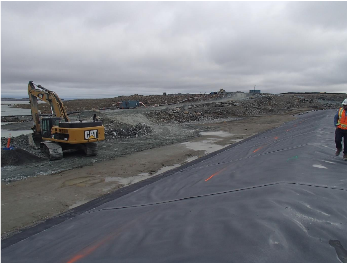
Photograph SD3-318: From Sta. 20+710/-24 m, looking SE. Placement of IV rockfill in the water up to El. 142m with an excavator from Sta. 20+785 m to 20+730 m, at the bottom of the upstream slope of SD3 to widen the rockfill layer and allow access to the erosion protection.
