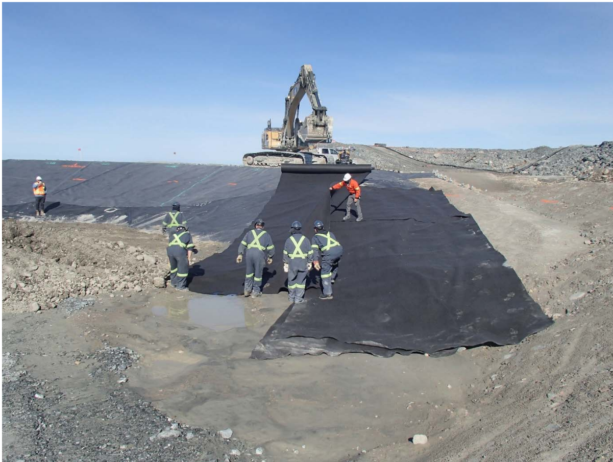
Photograph SD3-322: From Sta. 20+625/-63 m, looking W. Installation of two layers of geotextile on the upstream slope 3H:1V between El. 142 m and 143 m (approx.) from Sta. 20+610 m to 20+800 m.
