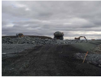
NCIS-128 (2018-07-28), looking NE from Sta. 1+680/-42 m (approx.). Placement of a 2 m thick (approx.) lift of UM rockfill from El. 152 m to El. 154 m (approx.) with a dozer from Sta. 1+830 m to 1+660 m (+8 m to -31 m) and profiling of the upstream slope (3H:1V) from El. 152 to 154 m with an excavator from Sta. 1+880 m to 1+780 m.
