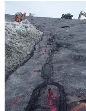
CD-1867 (2018-05-25), looking E from Sta. 40+680/-37 m. View of repair patches on the extrusion weld at the bottom of the panels.
