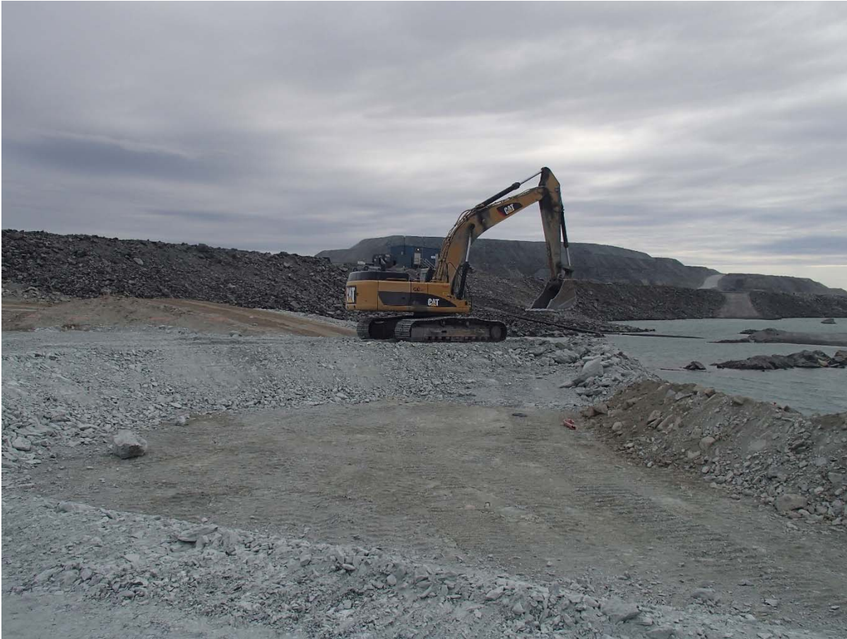
Photograph SD3-347: From Sta. 20+640/-41 m, looking W. Placement of a third 0.5 m thick lift of fine UM rockfill (0-500 mm) upstream of the low quality till (0-150mm) from El. 143 m to 143.5 m from Sta. 20+688 m to 20+619 m.
