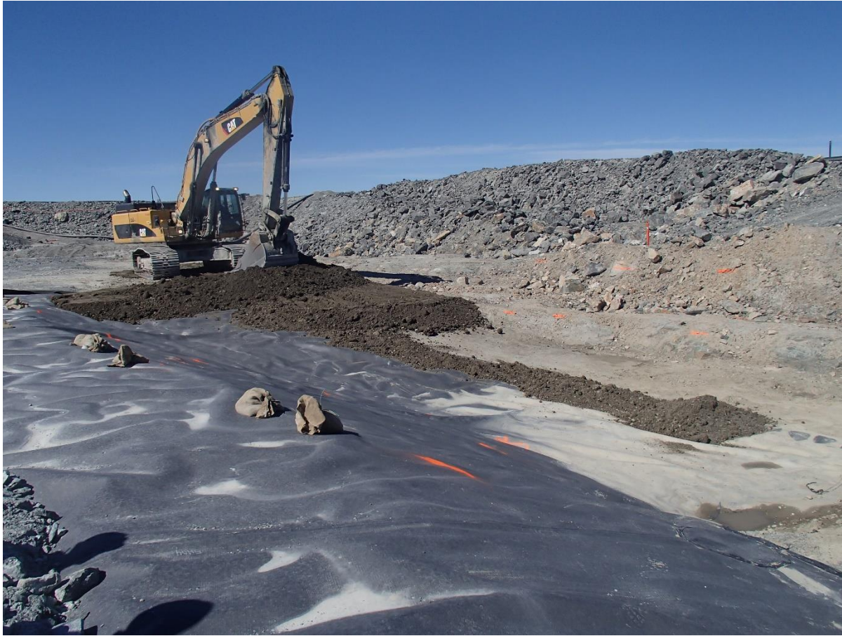
Photograph SD3-338: From Sta. 20+610/-43 m, looking NW. Placement of a first 0.5 m thick lift of compacted sieved till over the LLDPE geomembrane on the upstream toe liner tie-in with an excavator from Sta. 20+588 m to 20+599 m.
