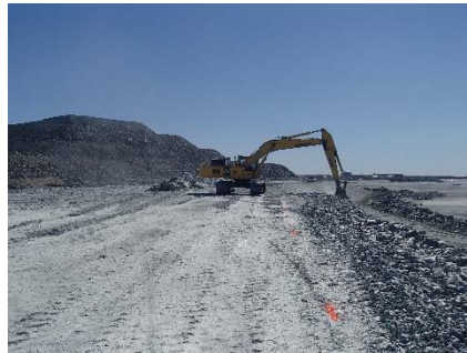
NCIS-095 (2018-07-16), looking S from Sta. 2+375/-18 m (approx.). Profiling of the upstream slope (3H:1V) from El. 152 to 154 m with an excavator from Sta. 2+545 m to 2+410 m.
