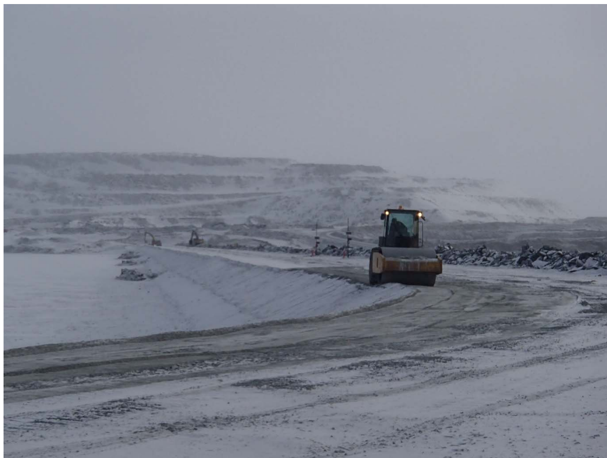
Photograph CD-1848: From Sta. 40+780/-15 m, looking N. Compaction of the fourth 0.5 m lift (approx.) of fine and coarse filters material at El. 145 m with a 10-tonne smooth-drum compactor with vibration (4 passes) from Sta 0+930 m to 40+730 m.
