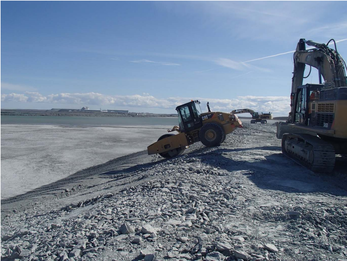
Photograph NCIS-099: From Sta. 1+180/-76 m (approx.), looking SE. Compaction of the 0.5 m lift (approx.) of coarse filter between El. 150 m and 152 m with a 10-tonne smooth-drum compactor with vibration (4 passes) in the upstream slope from Sta. 1+200 m to 1+170 m.
