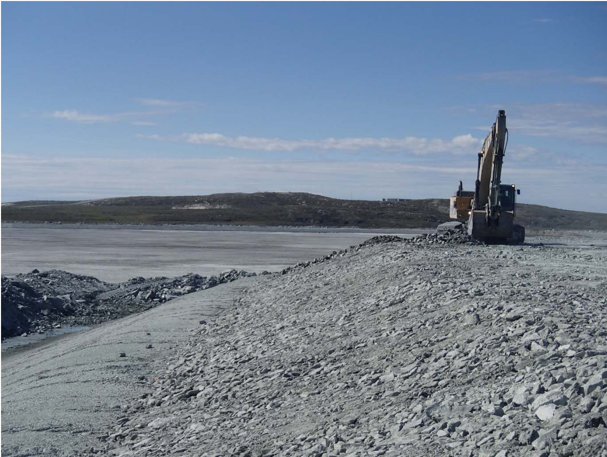
Photograph NCIS-102: From Sta. 2+680/-21 m (approx.), looking W. Placement of a 0.5 m thick lift of coarse filter in the upstream slope from El. 152 m to 154 m with an excavator from Sta. 2+575 m to 2+710 m and from Sta. 2+411 m to 2+460 m.
