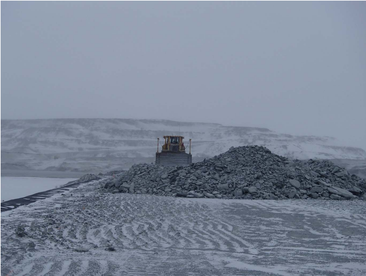
Photograph CD-1806: From Sta. 0+800/-27 m looking N. Placement a 2 m thick (approx.) lift of intermediate volcanic (IV) rockfill from El. 143 m to El. 145 m from approx. Sta. 0+710 to 0+760 m (o.s. -28 to 3 m).
