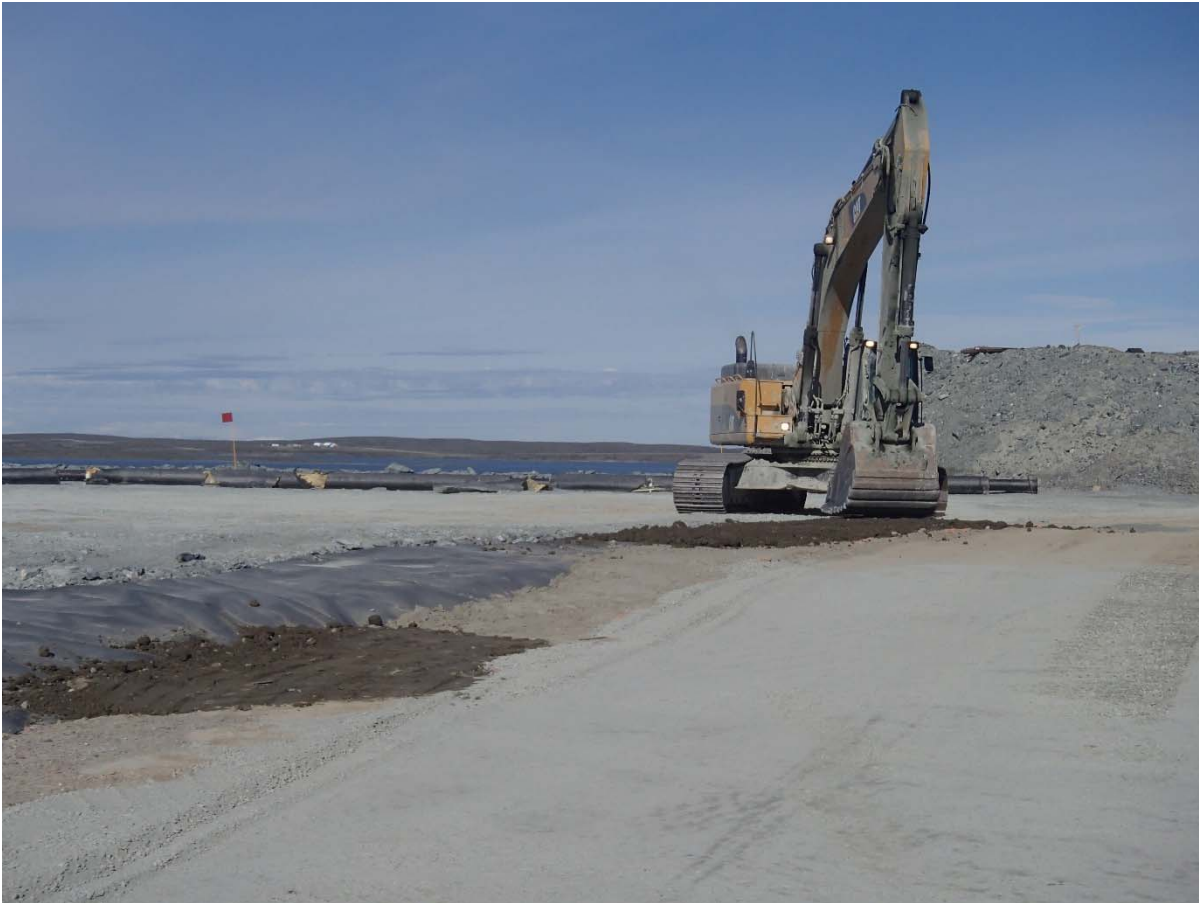
Photograph SD3-352: From Sta. 20+600/-59 m, looking SW. Corrections to the layer of compacted sieved till placed against the upstream slope from Sta. 20+599 m to 20+613 m.
