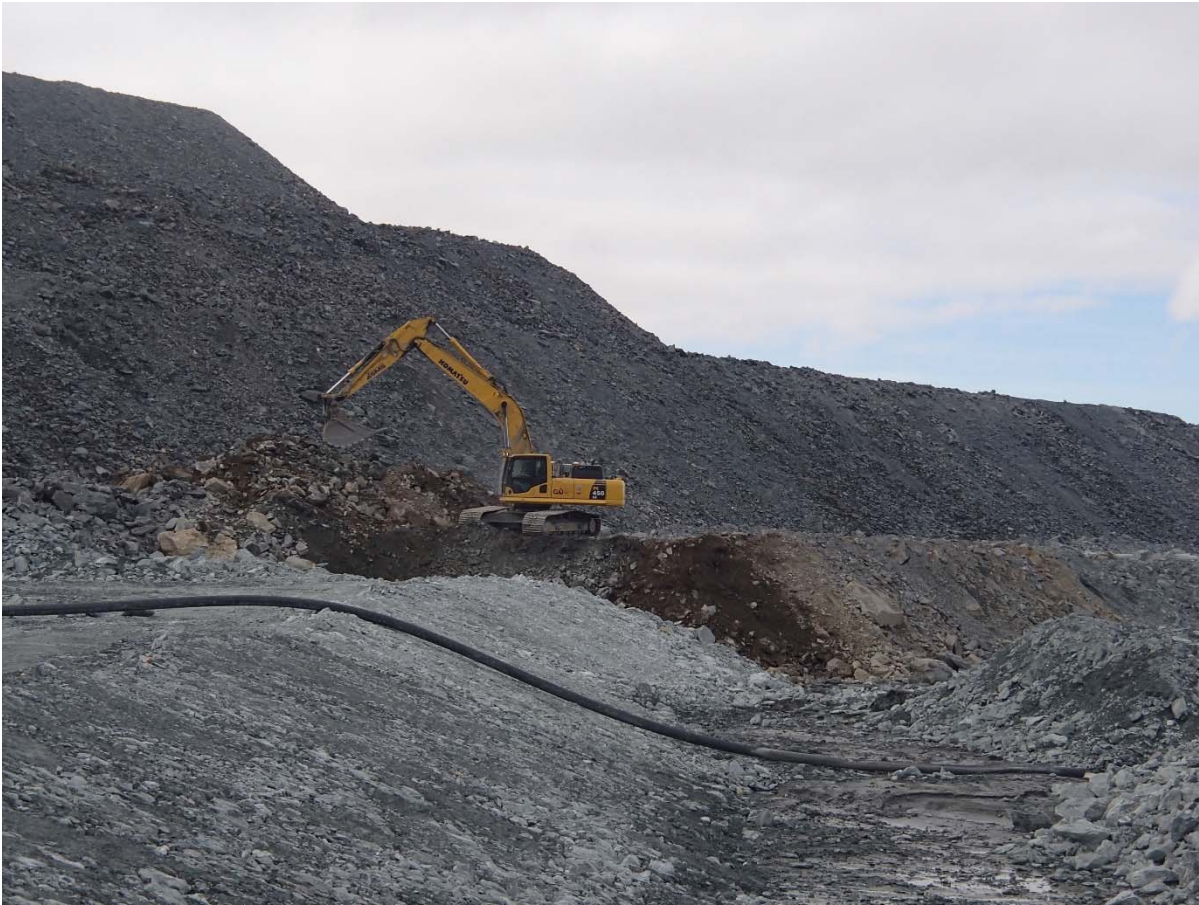
Photograph NCIS-046: From Sta. 2+680/-18 m (approx.), looking SE. Removal of till material mixed with the UM rockfill of the capping (about 1 to 2 m thick along the slope) with an excavator from Sta. 2+760 m to 2+850 m (offset -35 to -17 m).
