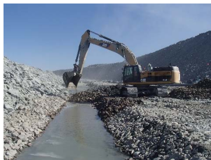
NCIS-125 (2018-07-27), looking NE from Sta. 3+050/+26 m (approx.). Corrections to the north sump: removal of approx. 0.5 m of tailing and till sieving reject material on the bottom of the excavation. The erosion protection material was replaced.
