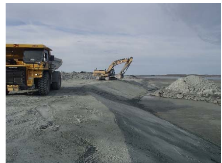
NCIS-081 (2018-07-06), looking SE from Sta. 2+975/-37 m (approx.). Placement of a 0.5 m thick lift of fine filter over the coarse filter in the upstream slope from El. 150 m to 152 m with an excavator from Sta. 1+300 m to 1+210 m and from Sta. 2+940 m to 3+120 m.
