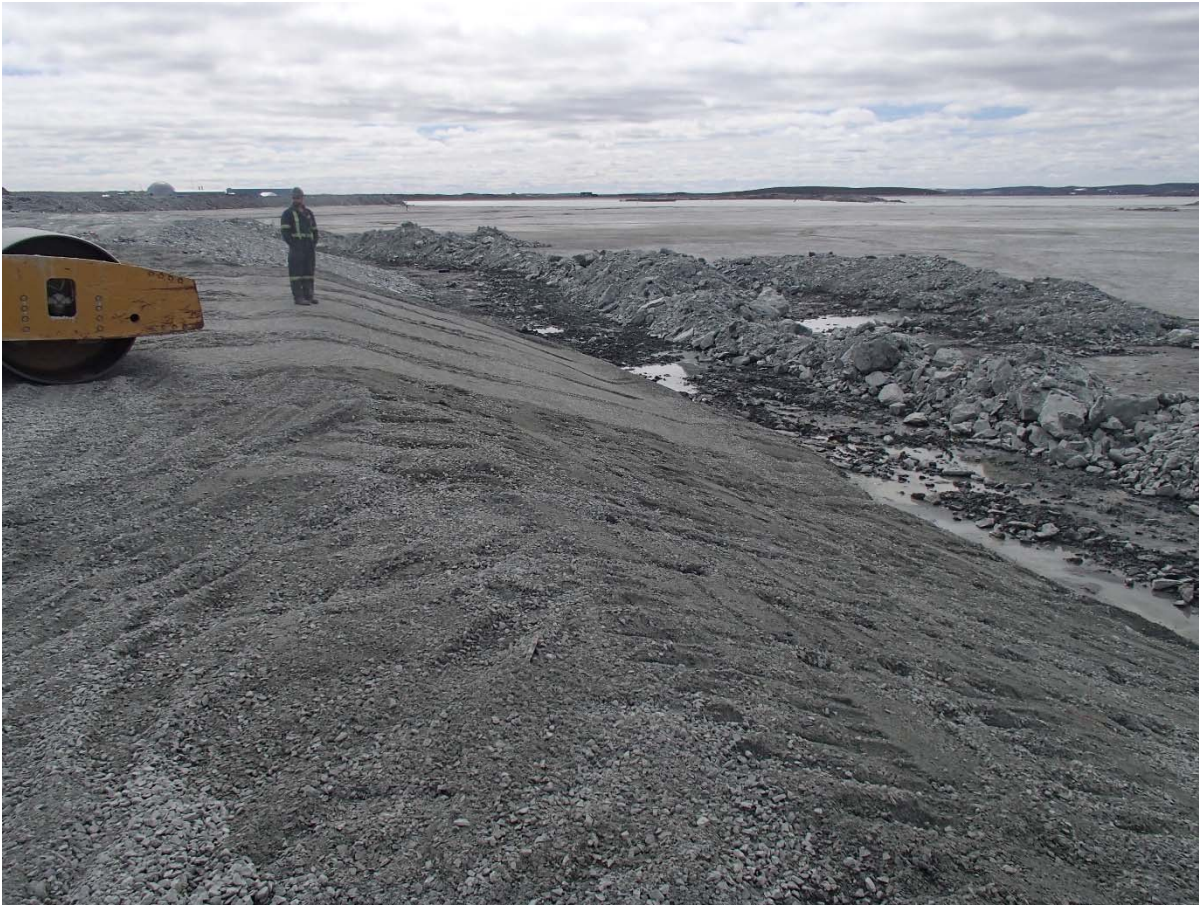
Photograph NCIS-038: From Sta. 2+510/-28 m (approx.), looking SE. Compaction of the 0.5 m lift (approx.) of fine filter between El. 150 and 152 m with a 10-tonne smooth-drum compactor (4 passes) in the upstream slope from Sta. 2+542 m to 2+475 m.
