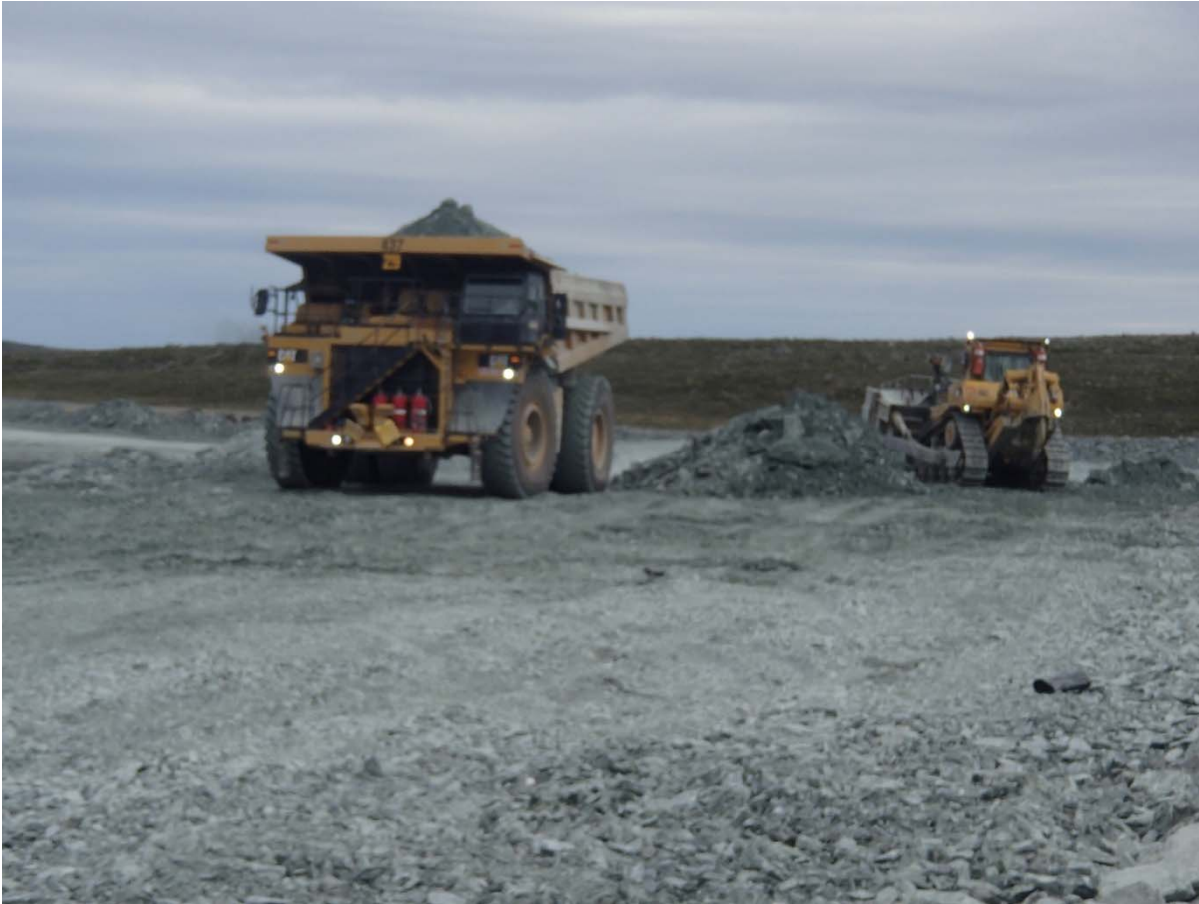
Photograph NCIS-096: From Sta 2+355/+9 m (approx.), looking N. Placement of a 2 m thick (approx.) lift of UM rockfill from El. 152 m to El. 154 m (approx.) with a dozer from Sta. 2+190 m to 2+103 m (+7 m to -22 m). The material is of good quality and is well graded.
