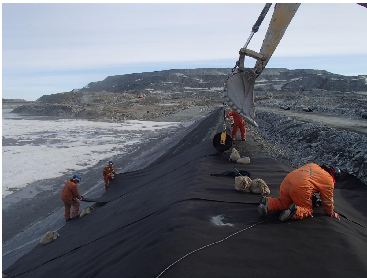
Photograph CD-1887: From Sta. 0+310/-26 m, looking N. Installation of the geotextile on the upstream slope 2H:1V between El. 143 m and 145 m from Sta. 0+320 m to 0+150 m.
