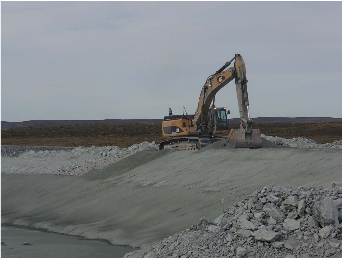
Photograph NCIS-136: From Sta. 1+800/-33 m (approx.), looking SW. Placement of a 0.5 m thick lift of fine filter in the upstream slope from El. 152 m to 154 m with an excavator from Sta. 1+700 m to 1+660 m.
