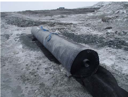
SD3-303 (2018-05-21), looking N from Sta. 20+780/-15 m. View of a LLDPE liner roll stored on geotextile.
