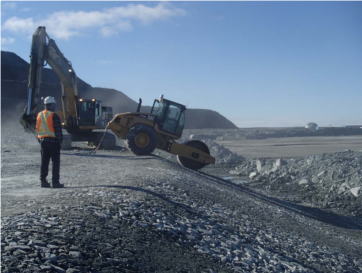
Photograph NCIS-054: From Sta. 2+580/-31 m (approx.), looking SE. Compaction of the 0.5 m lift (approx.) of coarse filter between El. 150 and 152 m with a 10-tonne smooth-drum compactor with vibration (4 passes) in the upstream slope from Sta. 2+560 m to 2+815 m.
