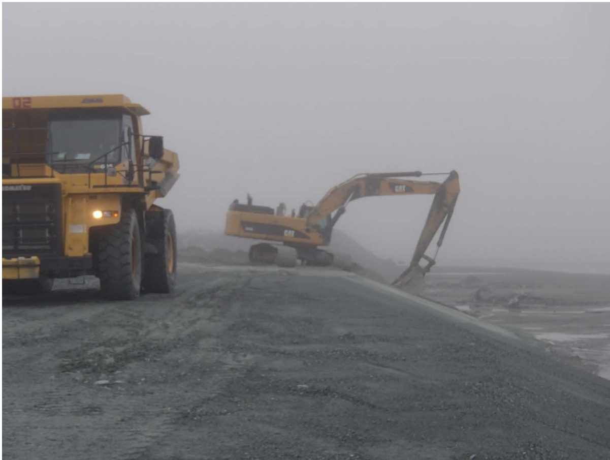
Photograph NCIS-082: From Sta 3+060/-33 m (approx.), looking S. Placement of a 0.5 m thick lift of fine filter over the coarse filter in the upstream slope from El. 150 m to 152 m with an excavator from Sta. 3+120 m to 3+160 m.
