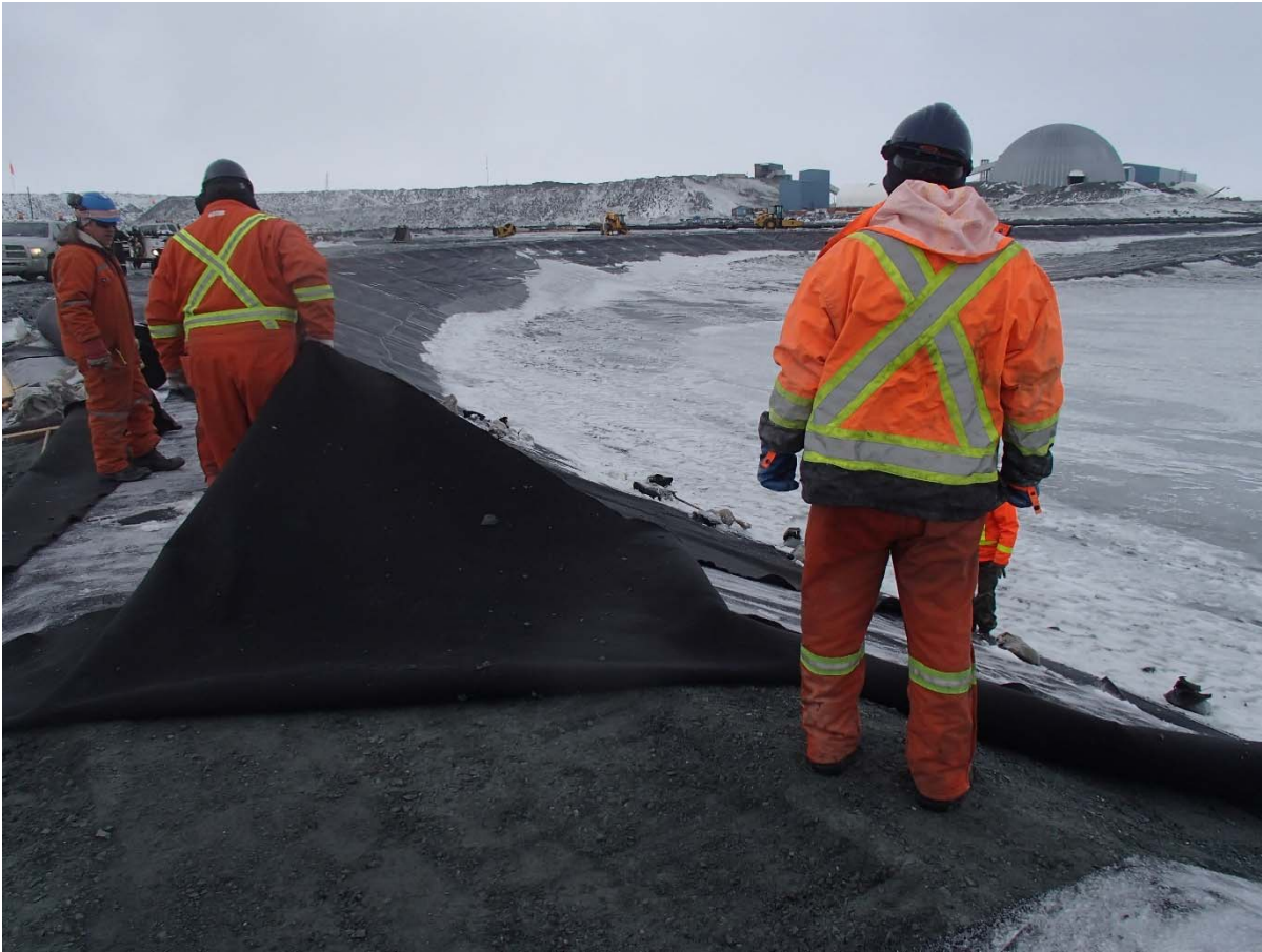
Photograph CD-1868: From Sta. 0+915/-24 m, looking S. Removal of the wet geotextile in place from Sta. 0+935 m to 0+900 m.
