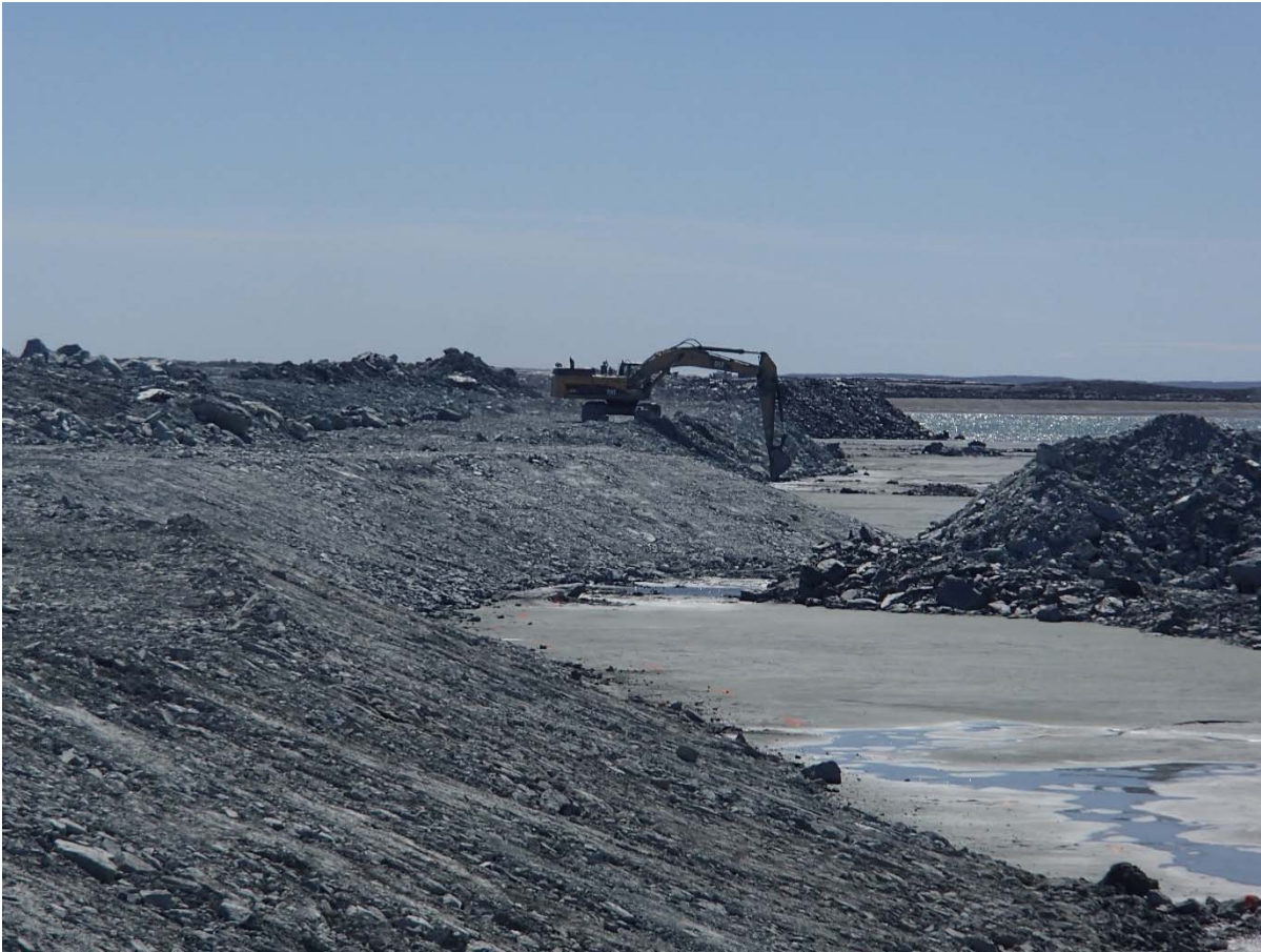
Photograph NCIS-072: From Sta. 2+790/-38 m (approx.), looking W. Profiling of the upstream slope (3H:1V) from El. 150 to 152 m with an excavator from Sta. 2+975 m to 3+070 m.
