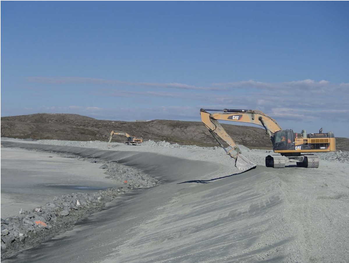
Photograph NCIS-113: From Sta. 2+220/-26 m (approx.), looking SW. Profiling of the upstream slope (3H:1V) from El. 152 to 154 m with an excavator from Sta. 2+000 m to 1+185 m and placement of a 0.5 m thick lift of fine filter in the upstream slope from El. 152 m to 154 m with an excavator from Sta. 2+300 m to 2+090 m.
