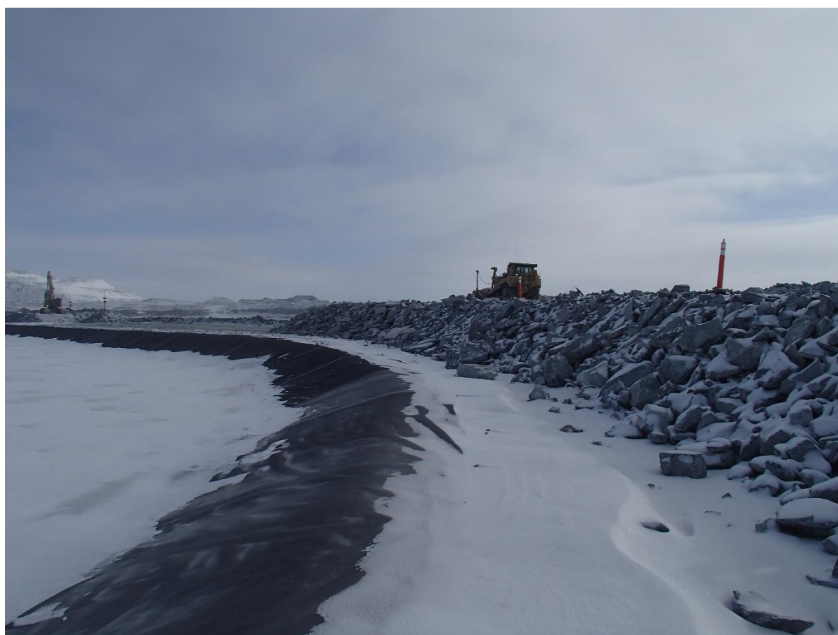
Photograph CD-1818: From Sta. 40+770/-25, looking NE. Placement of a 2 m thick (approx.) lift of intermediate volcanic (IV) rockfill from El. 143 m to El. 145 m from approx. Sta. 0+980 m to 0+880 m (o.s. -28 to -11 m).
