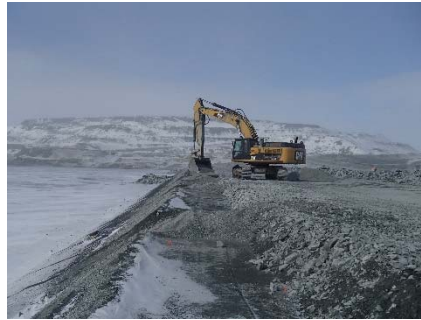
CD-1845 (2018-05-11), looking N from Sta. 0+660/-20 m. Profiling of the upstream slope (2H:1V) from El. 143 to 145 m with an excavator between Sta. 0+175 and 0+330 m and between Sta. 0+600 m and 0+715 m.
