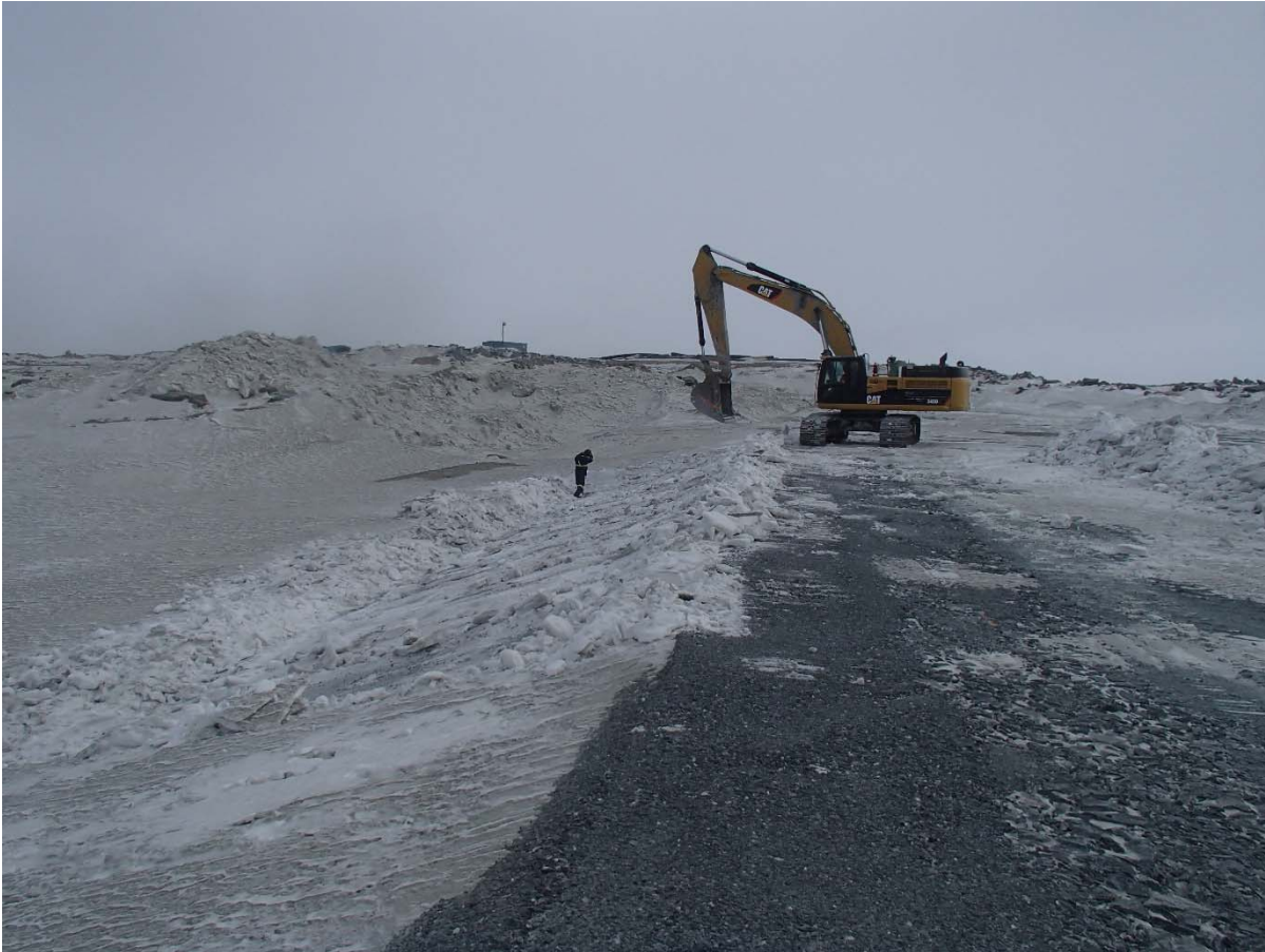
Photograph SD-297: From Sta. 20+730/-10 m, looking SE. Removal of snow on the upstream slope of SD3 with an excavator, from Sta. 20+640 to 20+760 m.
