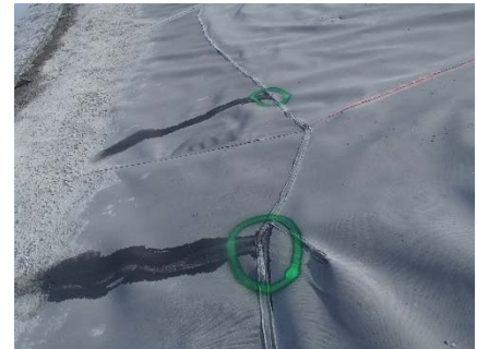
CD-1891 (2018-06-05), looking NE from Sta. 0+960/-28 m. View of leaking extrusion fillet seams before their repair on panel 816 and 818.
