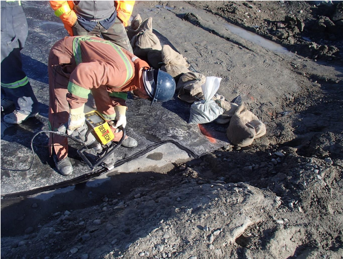
Photograph SD3-316: From Sta. 20+610/-45 m, looking NW. Repairs on the extrusion fillet seam between LLDPE panel 965 and the existing LLDPE panel at Sta. 20+600 m (approx.).
