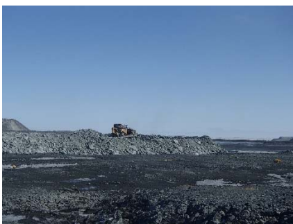
NCIS-025 (2018-06-01), looking SE from Sta. 1+475 m. Placement of a 2 m thick (approx.) lift of UM rockfill from El. 150 m to El. 152 m (approx.) with a dozer from Sta. 1+450 m to 1+390 m (o.s. unavailable). The material is of good quality and is well graded.
