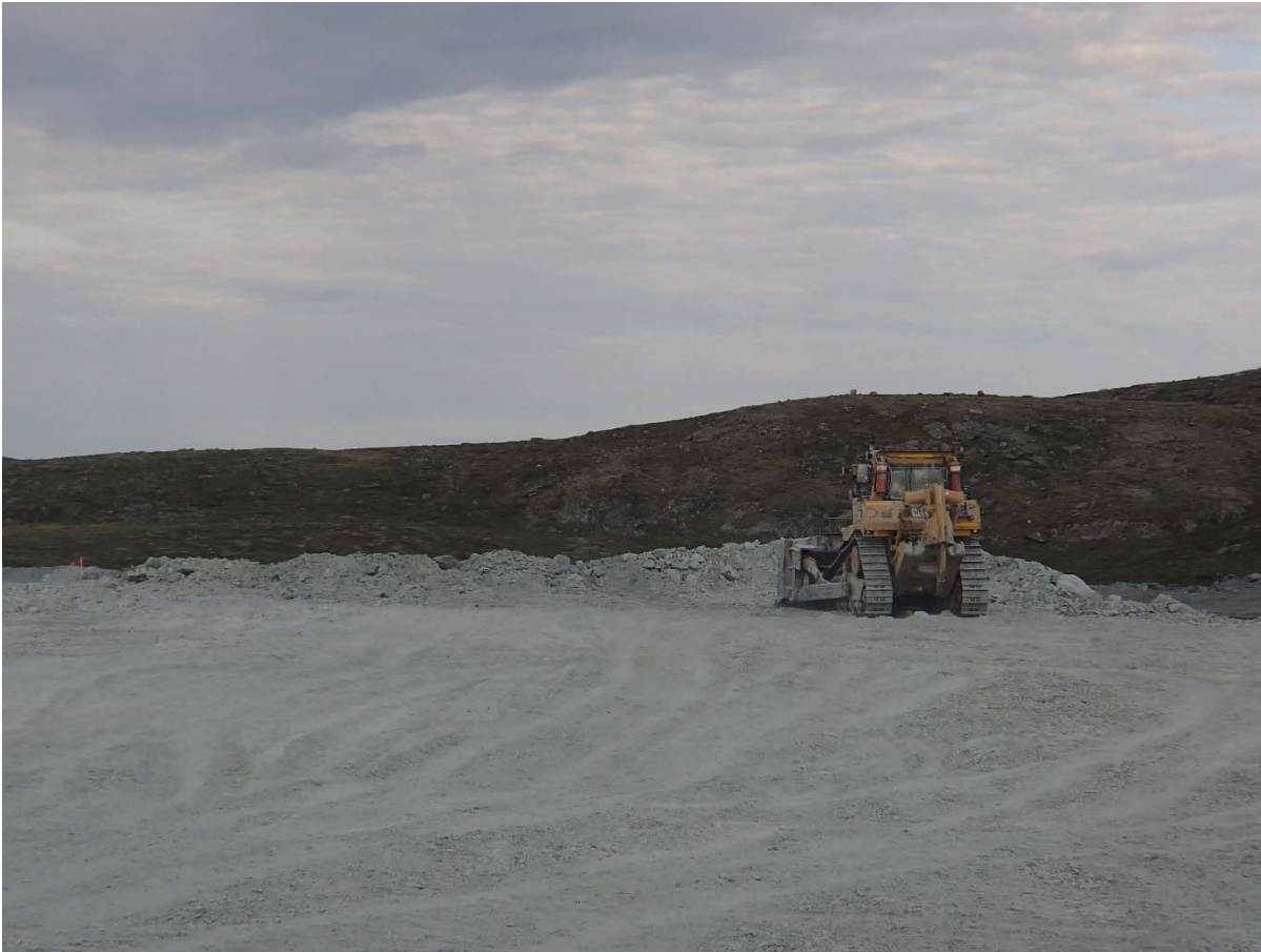
Photograph NCIS-122: From Sta. 1+960/-6 m (approx.), looking W. Placement of a 2 m thick (approx.) lift of UM rockfill from El. 152 m to El. 154 m (approx.) with a dozer from Sta. 1+830 m to 1+860 m (+8 m to -23 m).
