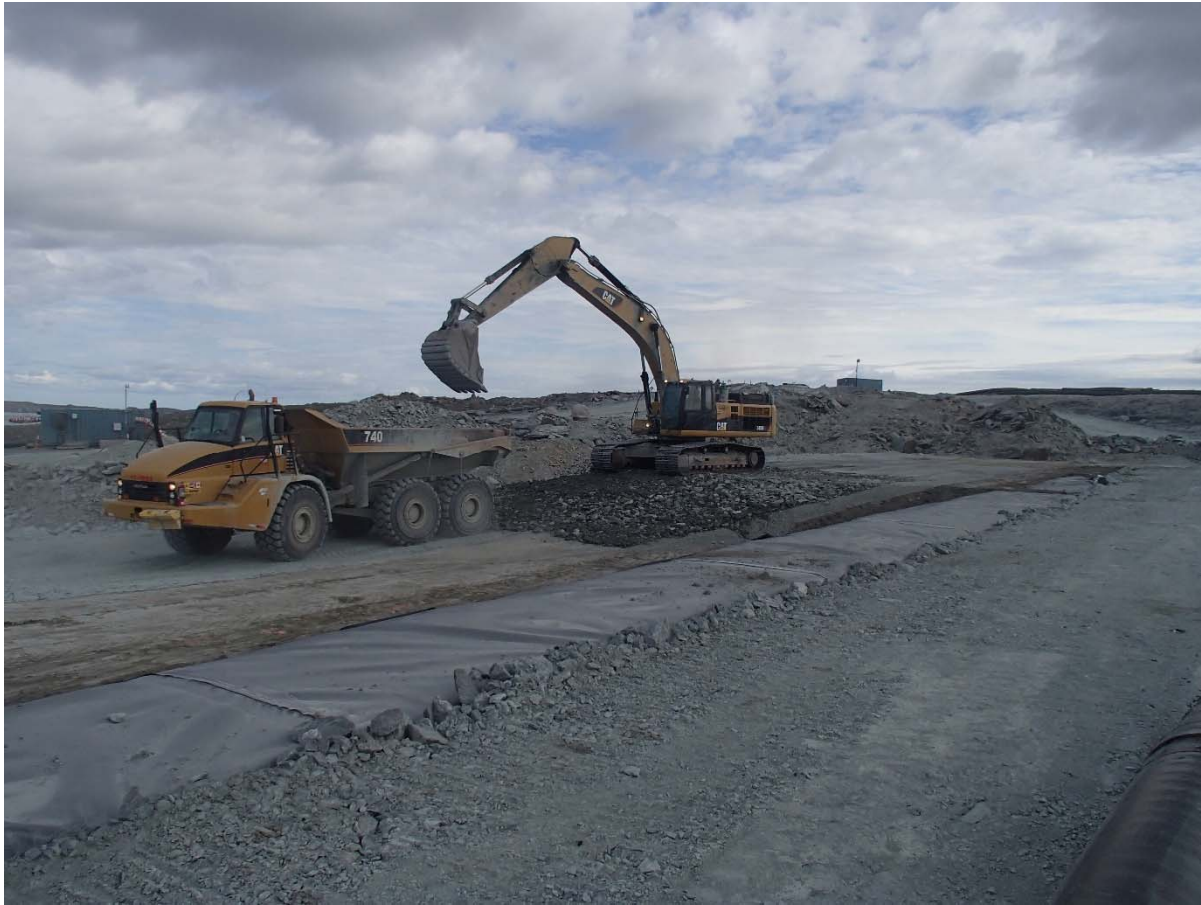
Photograph SD3-350: From Sta. 20+740/-24 m, looking SE. Placement of a 0.5 m thick lift of coarse filter on the top of the fine filter on the upstream toe liner tie-in with an excavator from Sta. 20+777 m to 20+807 m.
