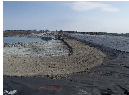
SD3-323 (2018-07-09), looking S from Sta. 20+610/-43 m. Placement of the first 0.5 m thick lift of low quality till (0-150 mm) from El. 142 m to 142.5 m from Sta. 20+610 m to 20+715 m.
