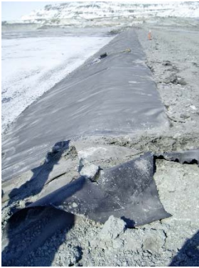
CD-1796 (2018-04-23), looking N from Sta. 0+650/-28 m. Damaged geomembrane near a deposition finger on Central Dike.
