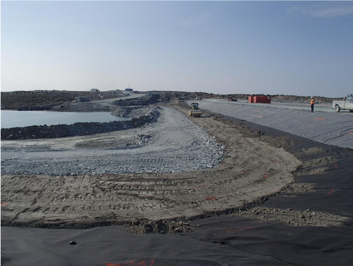
Photograph SD3-327: From Sta. 20+610/-43 m, looking S. Compaction of the 0.5 m lift of low quality till (0-150 mm) at El. 142.5 m with a 10-tonne smooth-drum compactor with vibration (4 passes) from Sta. 20+610 m to 20+615 m and from Sta. 20+635 m to 20+760 m.
