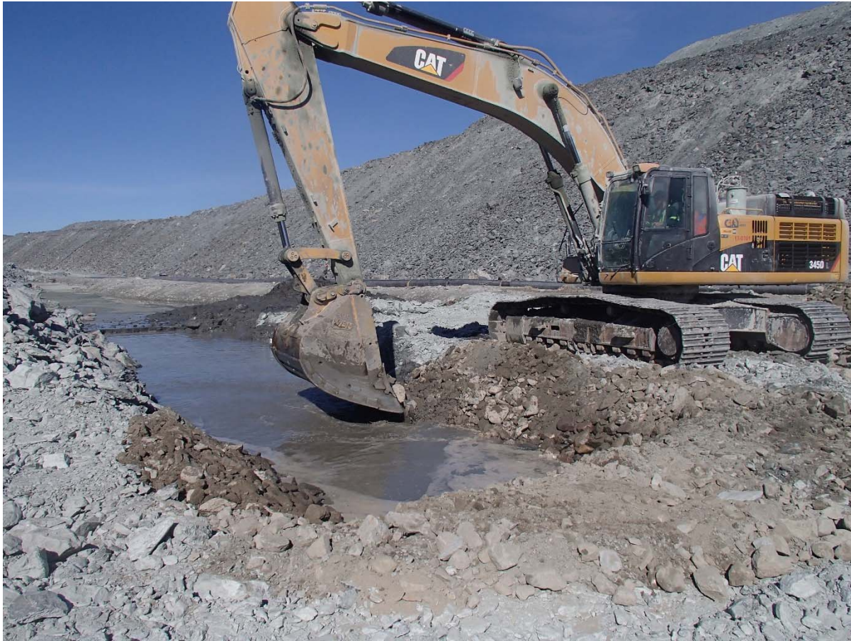
Photograph NCIS-121: From Sta.3+050/+26 m (approx.), looking NE. Placement of a 0.3 m thick (approx.) layer of till sieving reject material on the bottom and on the slopes of the sump.
