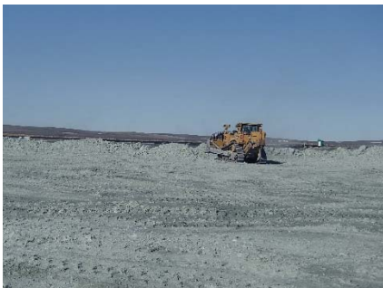
NCIS-052 (2018-06-27), looking SW from Sta. 1+120/-87 m. Placement of a 1.5 to 2 m thick (approx.) lift of UM rockfill from El. 148 m to El. 150 m (approx.) with a dozer from Sta. 1+115 m to 1+100 m (-107 m to -45 m).
