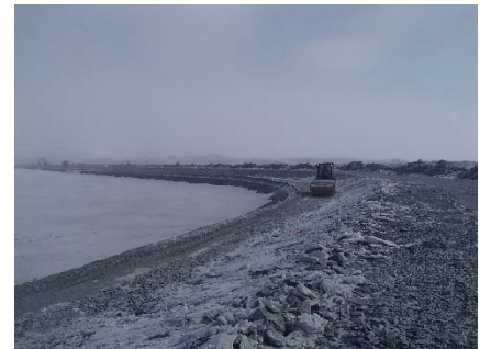
CD-1831 (2018-05-07), looking NE from Sta. 40+730/-24 m. Compaction of the 0.5 m lift (approx.) of fine and coarse filters material at El. 143.5 m with a 10-tonne smooth-drum compactor with vibration (6 passes) from Sta. 40+730 to 0+830 m.
