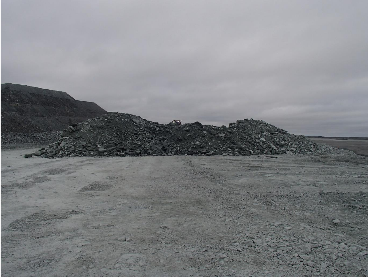
Photograph NCIS-090: From Sta 2+440/-1 m (approx.), looking SE. Placement of a 2 m thick (approx.) lift of UM rockfill from El. 152 m to El. 154 m (approx.) with a dozer from Sta. 2+455 m to 2+370 m (+4 m to -24 m).
