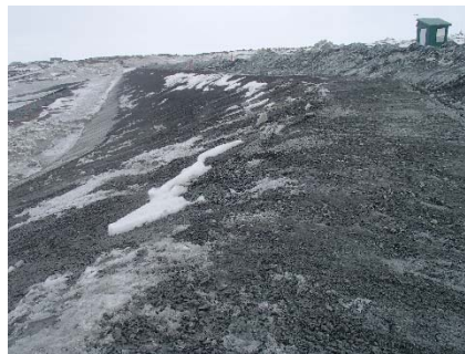
SD3-304 (2018-05-21), looking SE from Sta. 20+620/-36 m. Smoothing of the surface of the fine filter with an excavator on top of the upstream slope from Sta. 20+600 m to 20+780 m.
