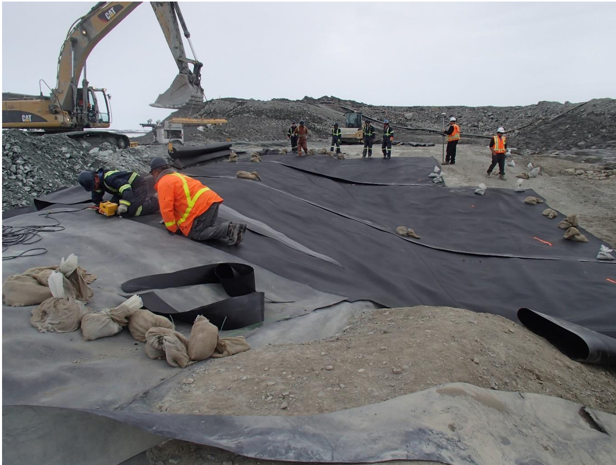
Photograph SD3-315: From Sta. 20+615/-46 m, looking W. Installation of the geotextile on the upstream slope 3H:1V between El. 143 m and 145 m from Sta. 20+593 m to 20+610 m and installation of the LLDPE liner on the upstream slope 3H:1V between El. 143 m and 145 m from Sta. 20+593 m to 20+610 m (panel numbers 965 to 967).
