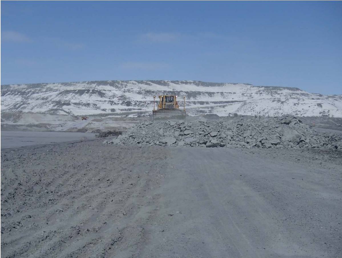
Photograph CD-1801: From Sta. 0+650/-10 m looking N. Placement a 2 m thick (approx.) lift of intermediate volcanic (IV) rockfill from El. 143 m to El. 145 m from 0+535 to 0+625m (o.s. -28 to -18 m).
