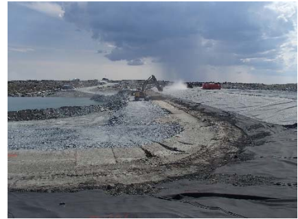
SD3-329 (2018-07-11), looking N from Sta. 20+820/-34 m. Placement of a 0.5 m thick lift of low quality till (0-150 mm) from El. 142.5 m to 143 m from Sta. 20+610 m to 20+760 m.
