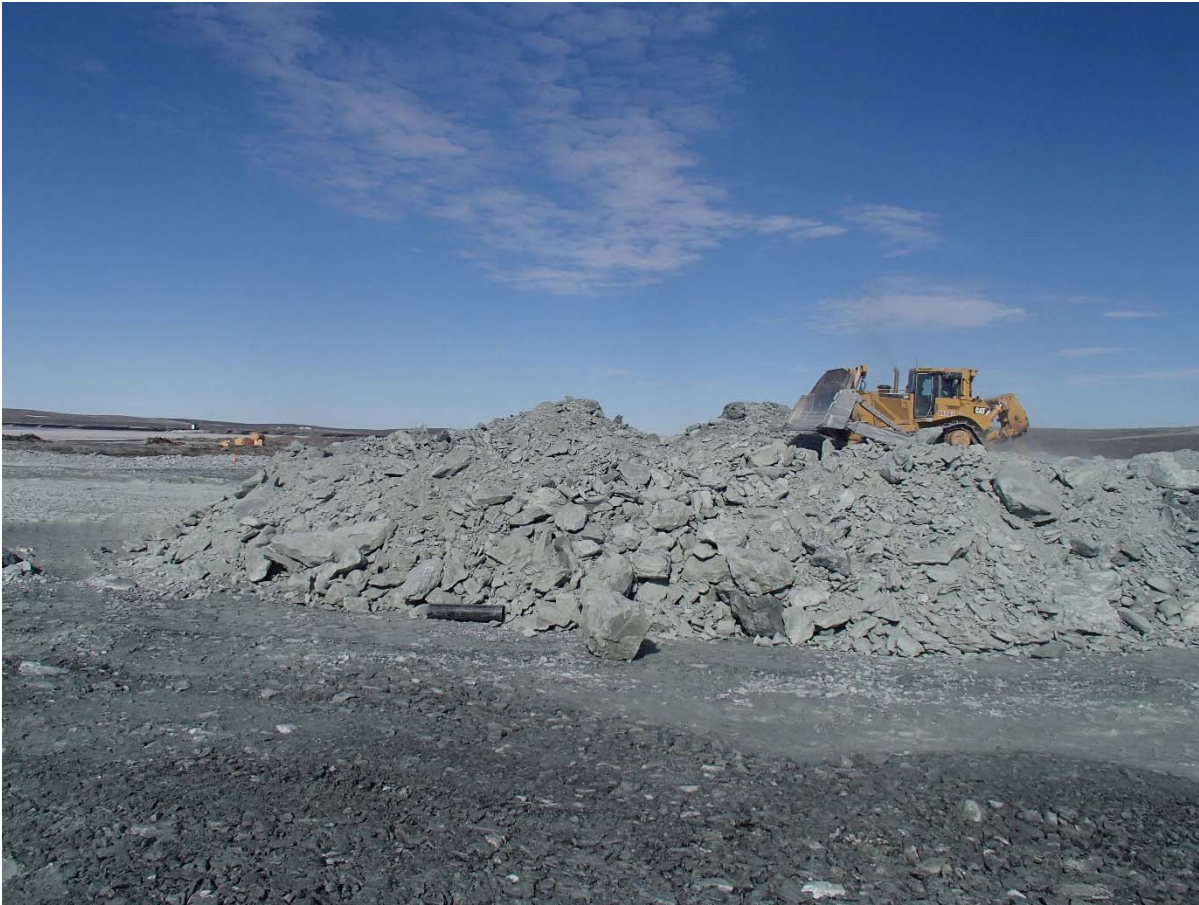
Photograph NCIS-064: From Sta. 1+200/-65 m (approx.), looking W. Placement of a 2 m thick (approx.) lift of UM rockfill from El. 150 m to El. 152 m (approx.) with a dozer from Sta. 1+320 m to 1+235 m (-65 m to -45 m). The material is of good quality and is well graded.
