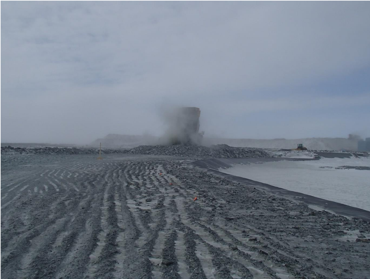
Photograph CD-1815: From Sta. 0+920/-25, looking S. Placement of a 2 m thick (approx.) lift of intermediate volcanic (IV) rockfill from El. 143 m to El. 145 m from approx. Sta. 40+740 to 0+980 m (o.s. -28 to -11 m).
