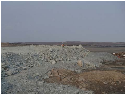
NCIS-085 (2018-07-09), looking SW from Sta. 1+150/-67 m (approx.). Placement of a 2 m thick (approx.) lift of UM rockfill from El. 150 m to El. 152 m (approx.) with a dozer from Sta. 1+130 m to 1+100 m (-55 m to -78 m).
