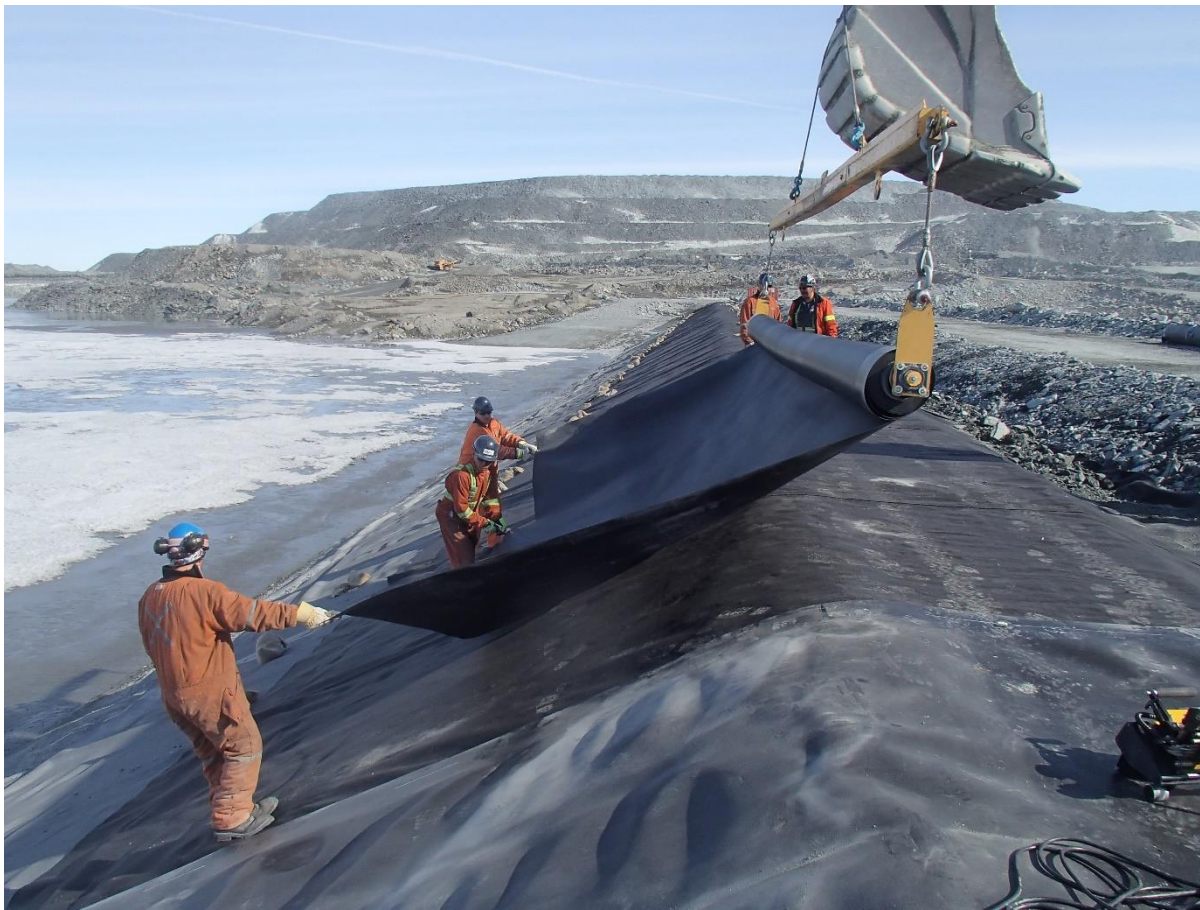
Photograph CD-1888: From Sta. 0+525/-26 m, looking N. Installation of the LLDPE liner on the upstream slope 2H:1V between El. 143 m and 145 m from Sta. 0+320 m to 0+150 m (panel numbers 911 to 933).
