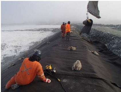
CD-1880 (2018-06-02), looking N from Sta. 0+600/-25 m. Installation of the geotextile on the upstream slope 2H:1V between El. 143 m and 145 m from Sta. 0+610 m to 0+480 m.
