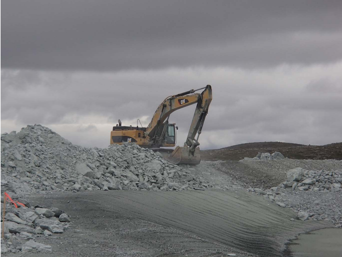
Photograph NCIS-134: From Sta. 1+630/-32 m (approx.), looking NE. Completion of the profiling of the upstream slope (3H:1V) from El. 152 to 154 m with an excavator from Sta. 1+700 m to 1+660 m.
