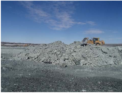
NCIS-064 (2018-06-30), looking W from Sta. 1+200/-65 m. Placement of a 2 m thick (approx.) lift of UM rockfill from El. 150 m to El. 152 m (approx.) with a dozer from Sta. 1+320 m to 1+235 m (-65 m to -45 m). The material is of good quality and is well graded.
