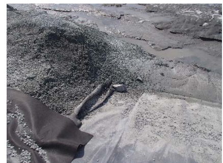
CD-1894 (2018-06-10), looking W from Sta. 0+800/-28 m. View of a block in direct contact with the LLDPE liner following the construction of the deposition fingers on Central Dike.
