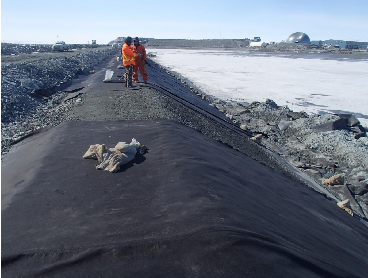
Photograph CD-1882: From Sta. 0+510/-25 m, looking S. View of the emplacement of the geotextile panel with a horizontal weld in the slope at Sta. 0+520 following its removal.
