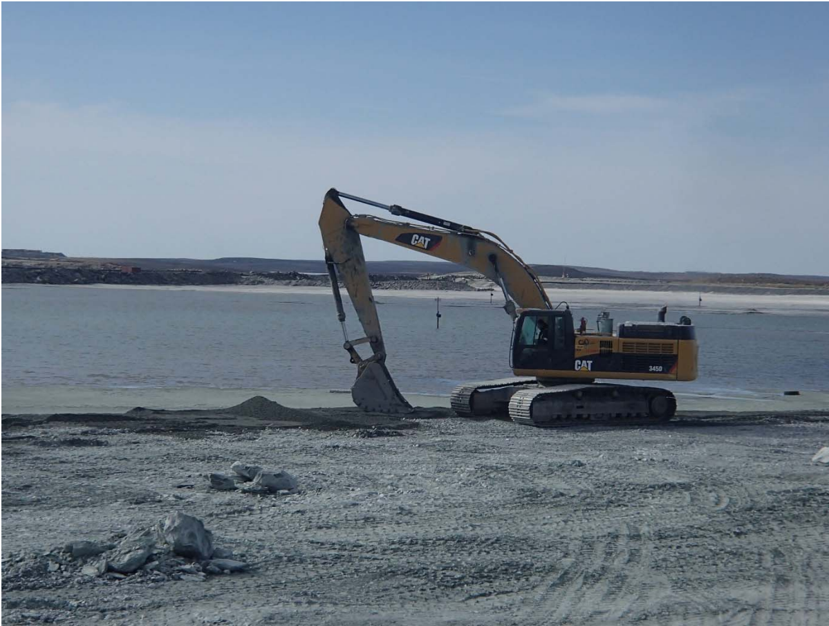
Photograph NCIS-068: From Sta. 1+150/-62 m (approx.), looking S. Placement of a 0.5 m thick lift of fine filter over the coarse filter in the upstream slope from El. 148 m to 150 m with an excavator from Sta. 1+180 m to 1+100 m.
