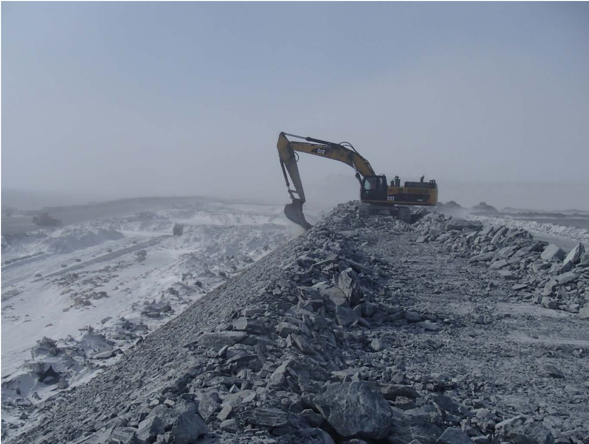
Photograph CD-1853: From Sta. 0+850/+3 m, looking S. Profiling of the downstream slope (1.5H:1V) from El. 143 to 145 m with an excavator between Sta. 0+835 m and 0+940 m.
