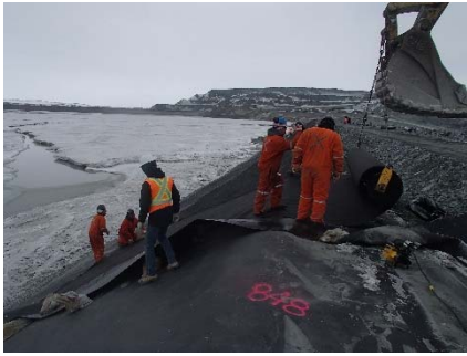
CD-1877 (2018-06-01), looking N from Sta. 0+745/-22 m. Installation of the geotextile on the upstream slope 2H:1V between El. 143 m and 145 m from Sta. 0+740 m to 0+610 m.
