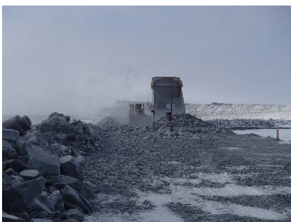
CD-1820 (2018-05-04), looking S from Sta. 0+790/-7 m. Placement of a 2 m thick (approx.) lift of intermediate volcanic (IV) rockfill from El. 143 m to El. 145 m from approx. Sta. 0+880 m to 0+830 m (o.s. -28 to -11 m).
