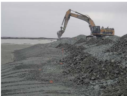
NCIS-079 (2018-07-05), looking SW from Sta. 1+280/-39 m. Placement of a 0.5 m thick lift of coarse filter in the upstream slope from El. 150 m to 152 m with an excavator from Sta. 1+300 m to 1+200 m.
