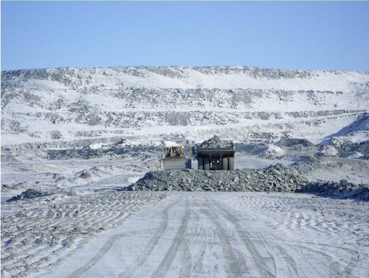
Photograph CD-1798: From Sta. 0+500/-15 m looking N. Placement of a 2 m thick (approx.) lift of intermediate volcanic (IV) rockfill from El. 143 m to El. 145 m from 0+340 to 0+435 m (o.s. -28 to -18 m).
