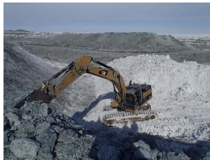
CD-1803 (2018-04-27), looking NE from Sta. 40+750/+27 m. Removal of snow to expose the foundation bedrock with an excavator between approx. Sta. 40+780 and 40+800 m (o.s. 7 to 10 m).
