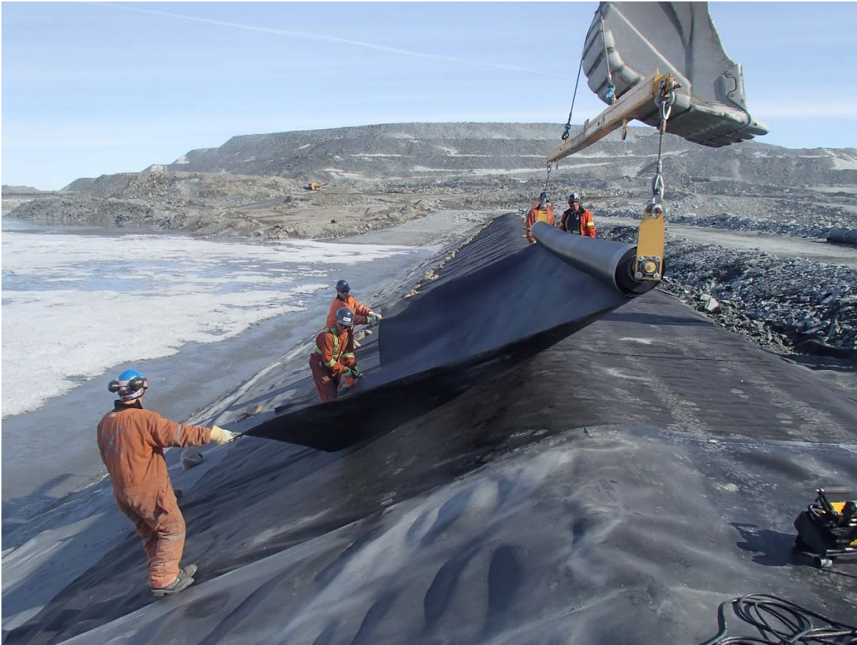
Photograph CD-1888: From Sta. 0+525/-26 m, looking N. Installation of the LLDPE liner on the upstream slope 2H:1V between El. 143 m and 145 m from Sta. 0+320 m to 0+150 m (panel numbers 911 to 933).
