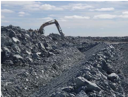
NCIS-130 (2018-07-28), looking S from Sta. 1+445/+16 m (approx.). Excavation of a 0.8 m (approx.) deep, 1 m wide shallow ditch in the rockfill capping with an excavator from Sta. 1+380 m to 1+300 m.
