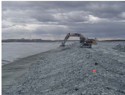
NCIS-077 (2018-07-04), looking S from Sta. 1+310/-32 m. Profiling of the upstream slope (3H:1V) from El. 150 m to 152 m with an excavator from Sta. 1+300 m to 1+175 m and from 3+070 m to 3+160 m.
