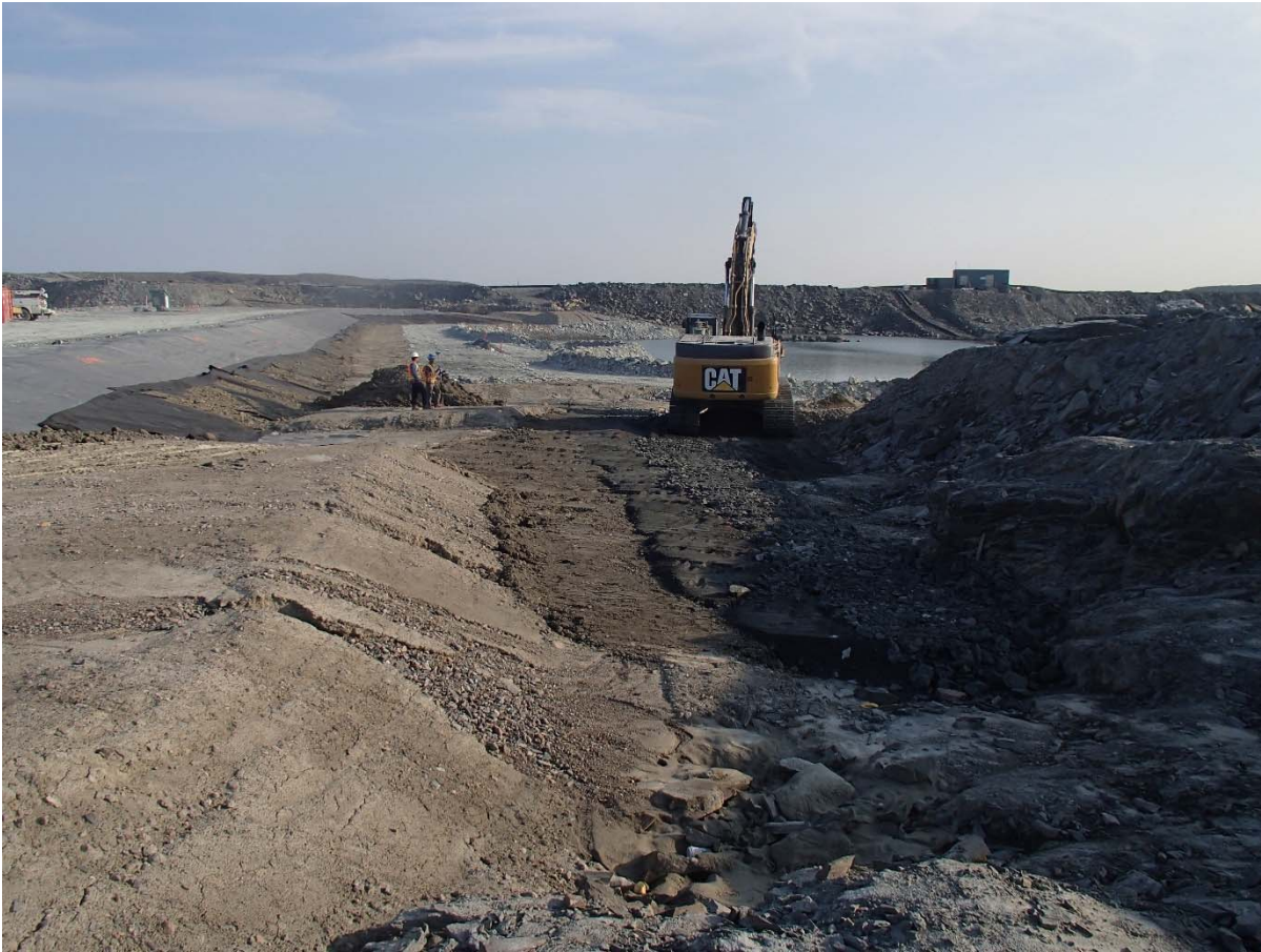
Photograph SD3-326: From Sta. 20+820/-34 m, looking N. Placement of the 0.5 m thick lift of low class till, fine filter, coarse filter and fine rockfill on the upstream slope of the upstream toe liner tie-in with an excavator from Sta. 20+780 to 20+810 m.
