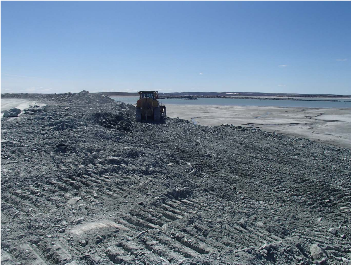
Photograph NCIS-057: From Sta. 3+010/-15 m (approx.), looking SW. Removing of UM rockfill material from the capping with a dozer to level the surface to El. 152 m from Sta. 2+980 m to 3+050 m (o.s. -30 to -20 m).
