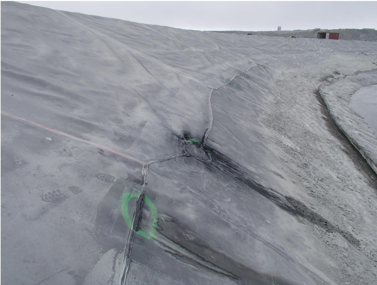
Photograph CD-1893: From Sta. 0+950/-27 m, looking SW. View of repair patches on the extrusion weld at the bottom of the panels 803, 807, 808, 810, 814, 815, 816 and 818.
