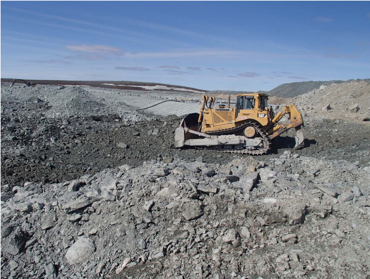
Photograph NCIS-049: From Sta. 2+870/-28 m (approx.), looking N. Removing of UM rockfill material from the capping with a dozer to level the surface to El. 150 m from Sta. 2+760 m to 2+850 m (offset -29 to -17 m).
