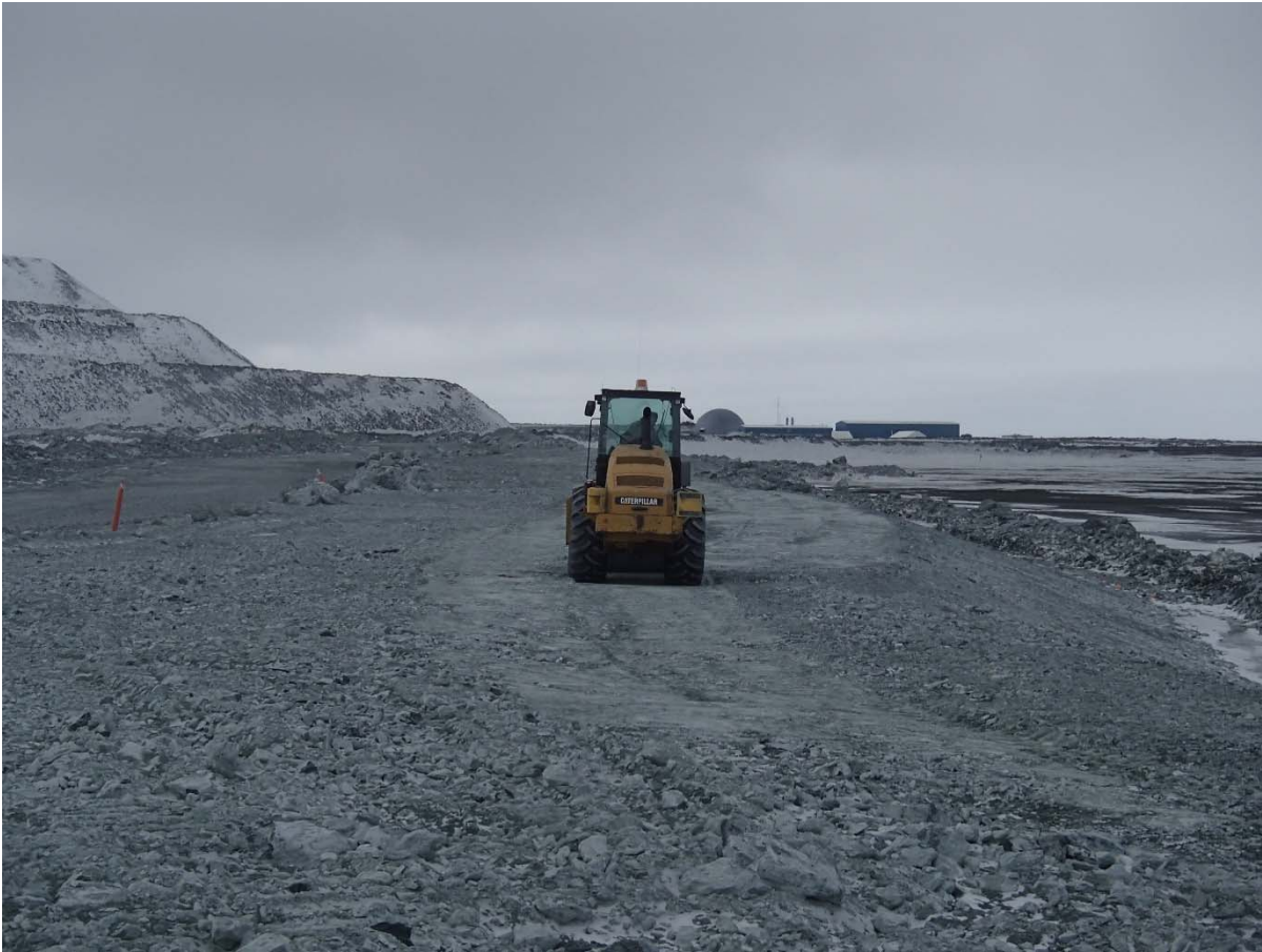
Photograph NCIS-022: From Sta. 2+245 m (approx.), looking SE. Compaction of the 2 m lift (approx.) of ultramafic (UM) rockfill at El. 152 m with a 10-tonne smooth-drum compactor with vibration (6 passes) between the haul truck traffic lane and the upstream slope from Sta. 2+625 to 1+625 m (offset unavailable).
