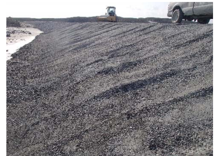
NCIS-087 (2018-07-11), looking W from Sta. 1+950/-34 m (approx.). Compaction of the 0.5 m lift (approx.) of fine filter between El. 150 and 152 m with a 10-tonne smooth-drum compactor (4 passes) in the upstream slope from Sta. 2+000 m to 1+930 m.
