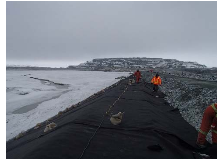
CD-1873 (2018-05-29), looking N from Sta. 0+760/-26 m. Installation of the geotextile on the upstream slope 2H:1V between El. 143 m and 145 m from Sta. 0+760 m to 0+740 m.
