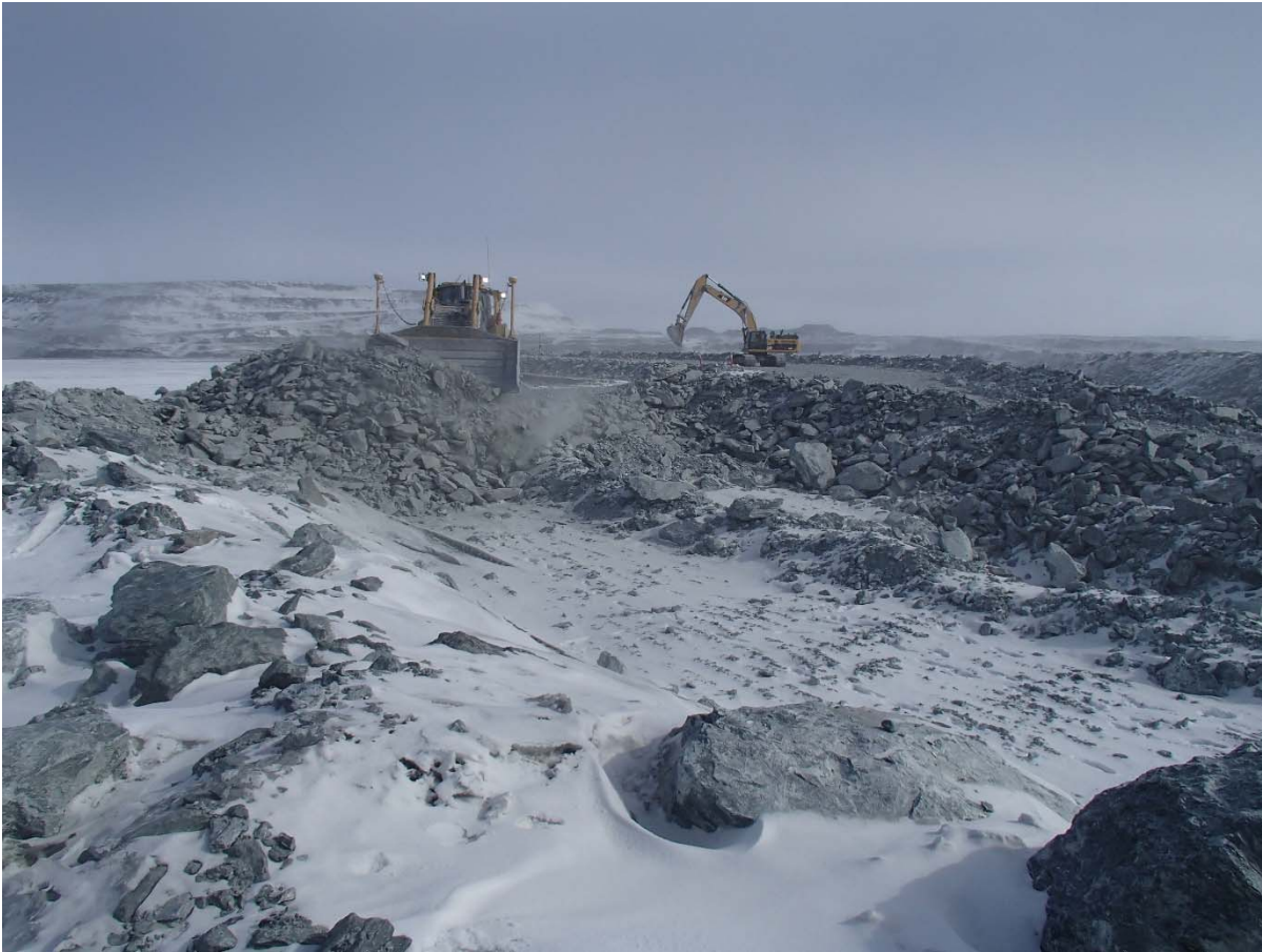
Photograph CD-1822: From Sta. 40+725/+7, looking N. Placement of two 2 m thick (approx.) lifts of intermediate volcanic (IV) rockfill from El. 141 m to El. 145 m from approx. Sta. 40+720 m to 40+750 m (o.s. -10 to +10 m) and profiling of the upstream slope (2H:1V) from El. 143 to 145 m with an excavator between Sta. 0+830 m and 0+980 m.
