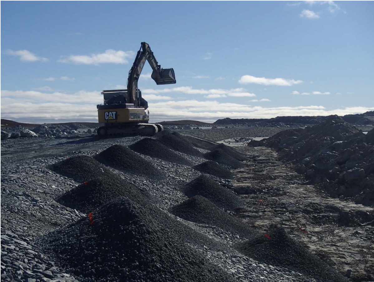
Photograph NCIS-055: From Sta. 1+730/-42 m (approx.), looking NE. Placement of a 0.5 m thick lift of fine filter over the coarse filter in the upstream slope from El. 150 m to 152 m with an excavator from Sta. 1+820 m to 1+595 m.
