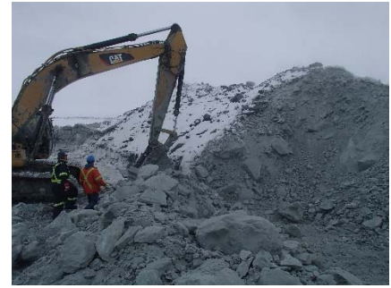
NCIS-003 (2018-05-19). Excavation of the snow-rich upstream toe material on an average width of 2 to 3 m with an excavator.
