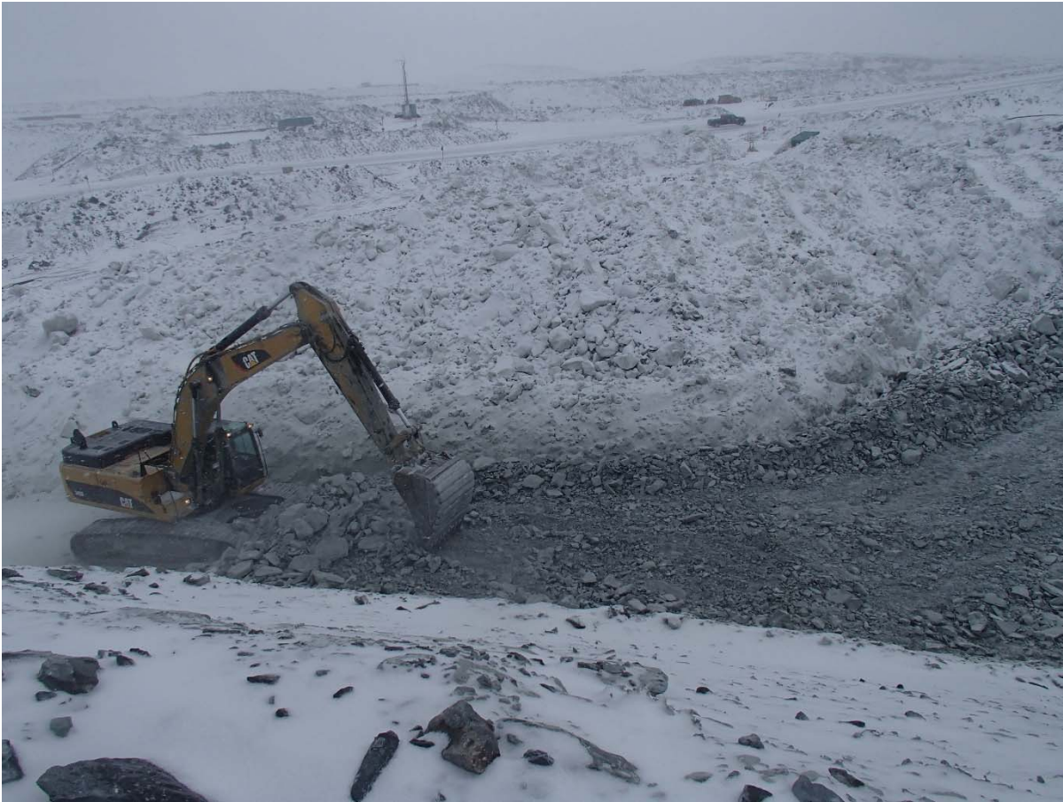
Photograph CD-1808: From Sta. 40+790/-14 m looking E. Placement a 1.5 m thick (approx.) lift of intermediate volcanic (IV) rockfill from approx. Sta. 40+780 to 40+805 m (o.s. -6 to 9 m).
