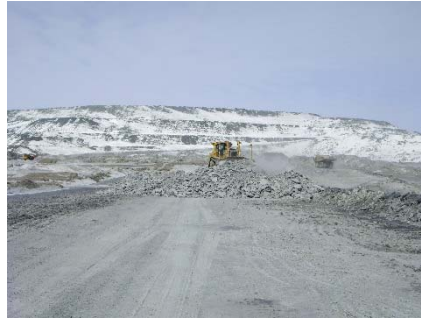
CD-1797 (2018-04-23), looking N from Sta. 0+380/-20 m. Placement a 2 m thick (approx.) lift of intermediate volcanic rockfill from El. 143 m to El. 145 m from 0+250 to 0+400 m (o.s. -28 to -18 m).
