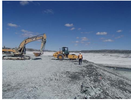
NCIS-065 (2018-06-30), looking NE from Sta. 1+140/-96 m. Compaction of the 0.5 m lift of coarse filter between El. 148 and 150 m with a 10-tonne smooth-drum compactor with vibration (4 passes) in the upstream slope from Sta. 1+270 m to 1+100 m.
