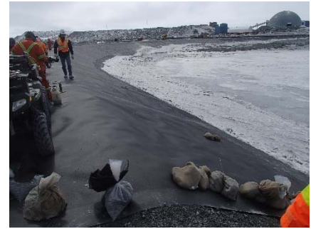
CD-1870 (2018-05-27), looking S from Sta. 0+900/-26 m. Installation of the LLDPE liner on the upstream slope 2H:1V between El. 143 m and 145 m from Sta. 0+935 m to 0+900 m (panel numbers 820 to 823).
