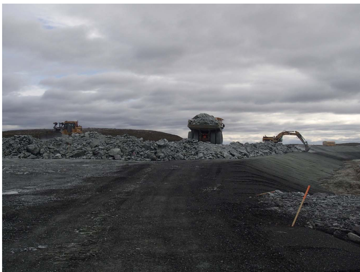
Photograph NCIS-128: From Sta. 1+680/-42 m (approx.), looking NE. Placement of a 2 m thick (approx.) lift of UM rockfill from El. 152 m to El. 154 m (approx.) with a dozer from Sta. 1+830 m to 1+660 m (+8 m to -31 m) and profiling of the upstream slope (3H:1V) from El. 152 to 154 m with an excavator from Sta. 1+880 m to 1+780 m.
