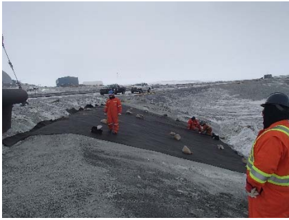
CD-1859 (2018-05-22), looking SW from Sta. 40+780/-38 m. Installation of the geotextile on the upstream slope 3H:1V (SD5 side) to 2H:1V (Central Dike side) between El. 143 m and 145 m from Sta. 40+640 m to 0+830 m.
