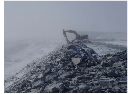
CD-1825 (2018-05-05), looking S from Sta. 0+430/+9 m. Profiling of the downstream slope (1.5H:1V) from El. 143 to 145 m with an excavator between Sta. 0+330 m and 0+440 m and between Sta. 0+530 m and 0+745 m.
