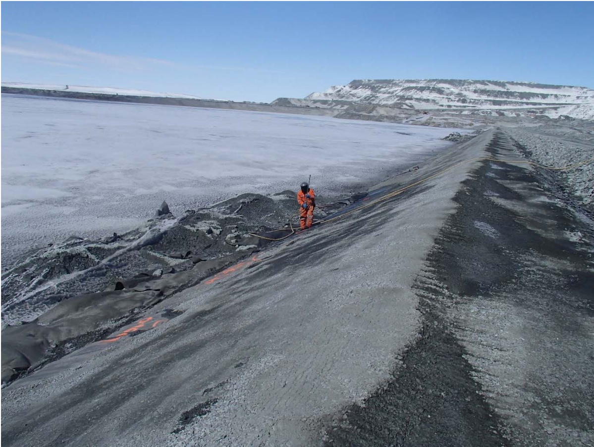
Photograph CD-1586: From Sta. 0+670/-24 m, looking N. Clean-up of the fine filter placed against the slope at the deposition finger at approx. Sta. 0+670 m with pressurized air stream to expose 1 m of LLDPE liner, in preparation for the new liner installation.
