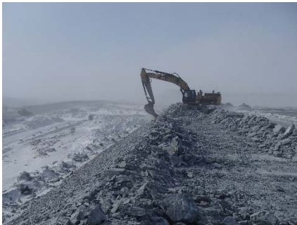
CD-1853 (2018-05-14), looking S from Sta. 0+850/+3 m. Profiling of the downstream slope (1.5H:1V) from El. 143 to 145 m with an excavator between Sta. 0+835 m and 0+940.
