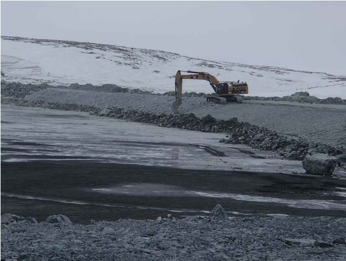
Photograph NCIS-017: From Sta. 2+290 m (approx.), looking SW. Profiling of the upstream slope (3H:1V) from El. 150 to 152 m with an excavator from Sta. 2+138 m to 1+989 m.
