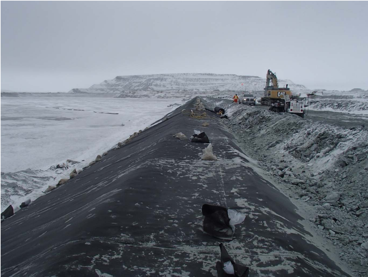
Photograph CD-1860: From Sta. 0+790/-26 m, looking N. Installation of the geotextile on the upstream slope 2H:1V between El. 143 m and 145 m from Sta. 0+830 m to 0+750 m.
