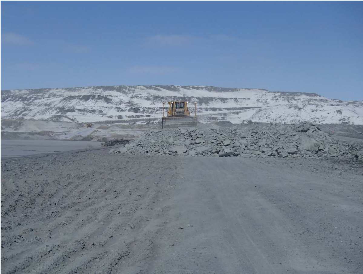
Photograph CD-1801: From Sta. 0+650/-10 m looking N. Placement of a 2 m thick (approx.) lift of intermediate volcanic (IV) rockfill from El. 143 m to El. 145 m from 0+535 to 0+625m (o.s. -28 to -18 m).
