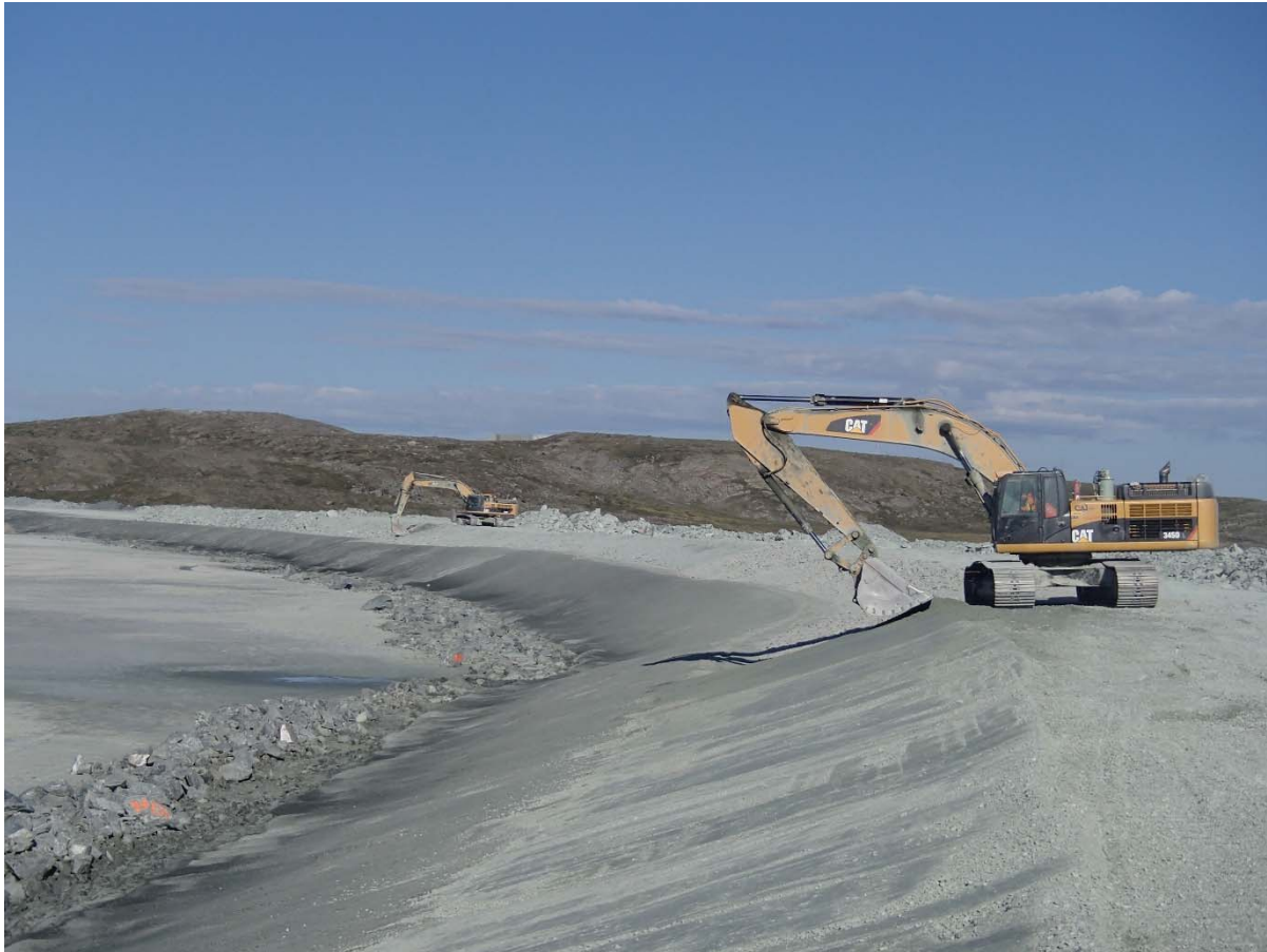
Photograph NCIS-113: From Sta. 2+220/-26 m (approx.), looking SW. Profiling of the upstream slope (3H:1V) from El. 152 to 154 m with an excavator from Sta. 2+000 m to 1+185 m and placement of a 0.5 m thick lift of fine filter in the upstream slope from El. 152 m to 154 m with an excavator from Sta. 2+300 m to 2+090 m.
