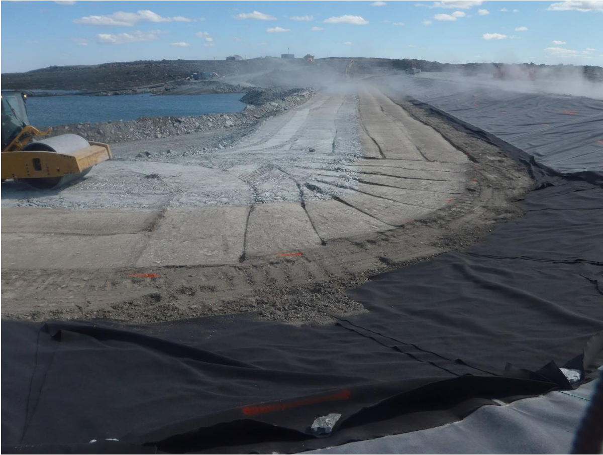
Photograph SD3-331: From Sta. 20+610/-43 m, looking S. Compaction of the 0.5 m lift of low quality till (0-150 mm) at El. 143 m with a 10-tonne smooth-drum compactor with vibration (4 passes) from Sta. 20+610 m to 20+760 m.
