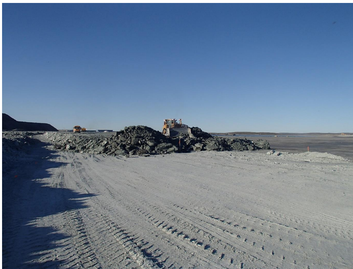
Photograph NCIS-093: From Sta 2+260/+12 m (approx.), looking S. Placement of a 2 m thick (approx.) lift of UM rockfill from El. 152 m to El. 154 m (approx.) with a dozer from Sta. 2+290 m to 2+280 m (+9 m to -22 m).
