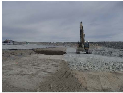
SD3-345 (2018-07-17), looking NW from Sta. 20+760/-42 m. Placement of a fourth 0.5 m thick lift of low quality till (0-150 mm) from El. 143 m to 143.5 m from Sta. 20+619 m to 20+777 m.
