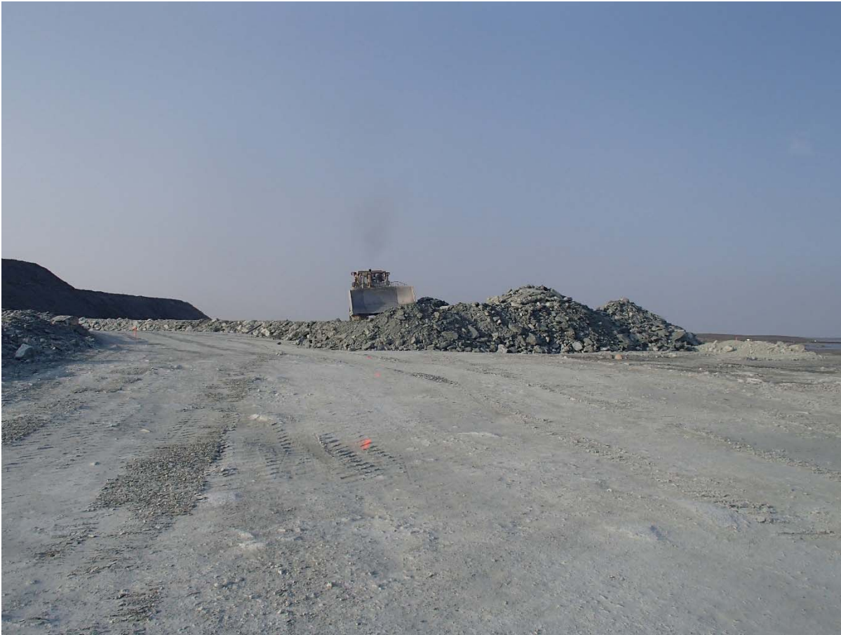
Photograph NCIS-089: From Sta 2+525/+4 m (approx.), looking S. Placement of a 2 m thick (approx.) lift of UM rockfill from El. 152 m to El. 154 m (approx.) with a dozer from Sta. 2+605 m to 2+455 m (+3 m to -23 m).
