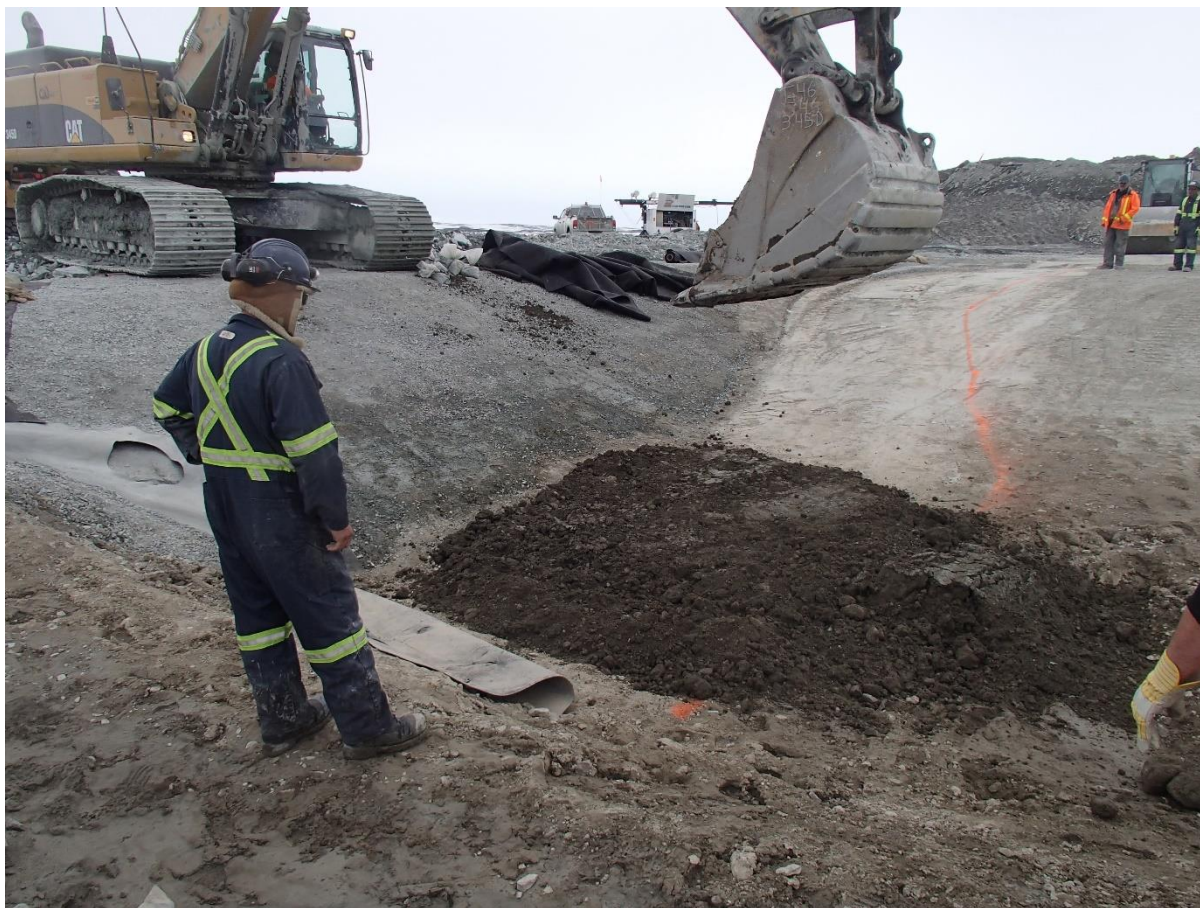
Photograph SD3-312: From Sta. 20+610/-48 m, looking W. Placement of a 0.15 m thick lift of compacted sieved till from Sta. 20+596.4 m to 20+601.6 m (o.s. -42.6 to -46.3 m) to fill the depression in the compacted sieved till layer.
