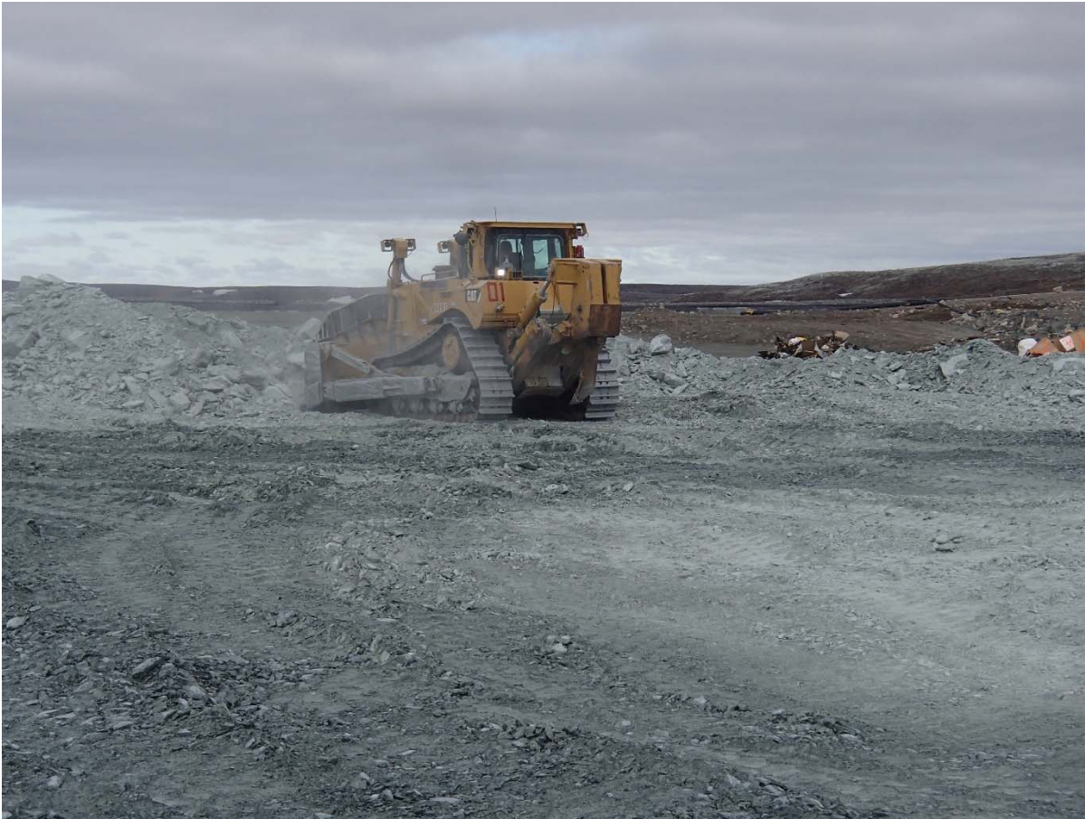
Photograph NCIS-048: From Sta. 1+120/-92 m (approx.), looking SW. Placement of a 1.5 to 2 m thick (approx.) lift of UM rockfill from El. 148 m to El. 150 m (approx.) with a dozer from Sta. 1+125 m to 1+115 m (-92 m to -47 m). The material is of good quality and is well graded.
