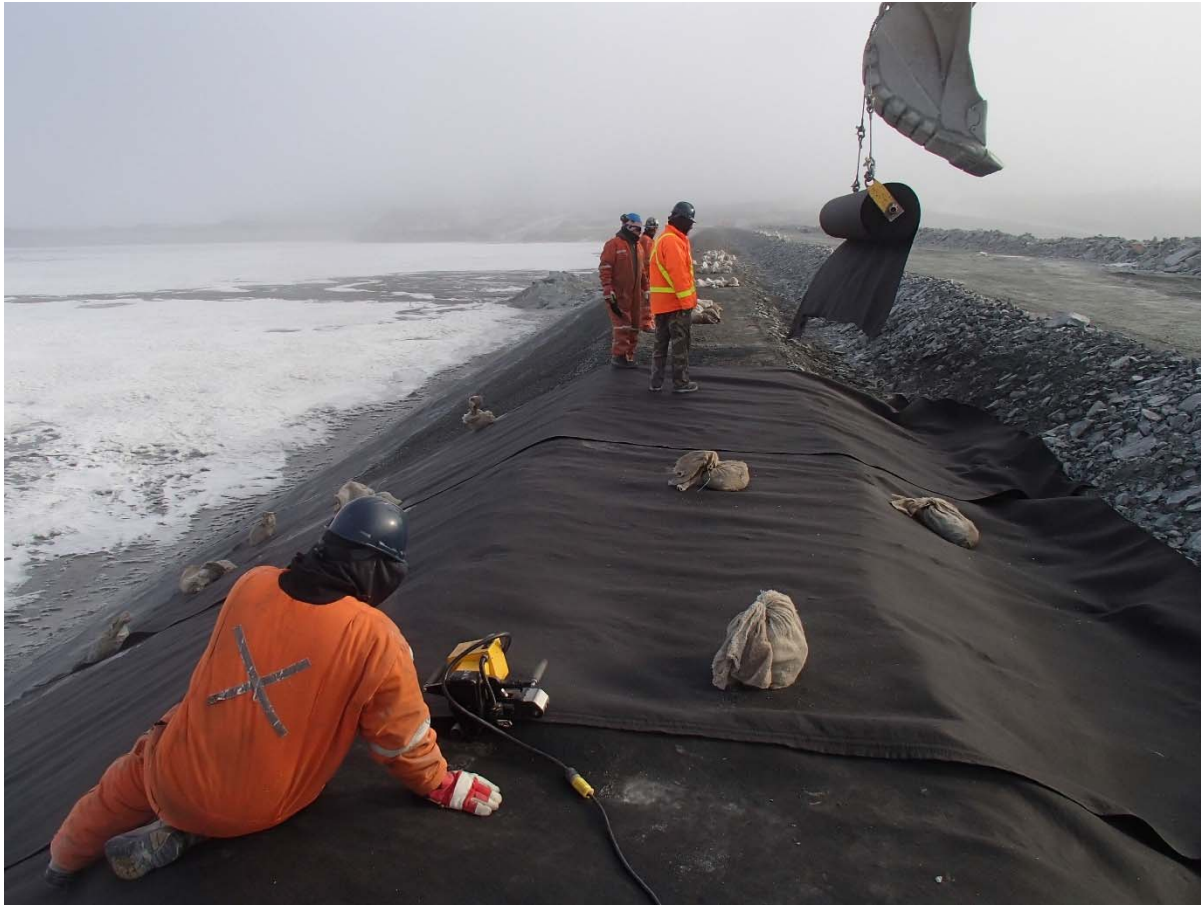
Photograph CD-1880: From Sta. 0+600/-25 m, looking N. Installation of the geotextile on the upstream slope 2H:1V between El. 143 m and 145 m from Sta. 0+610 m to 0+480 m.
