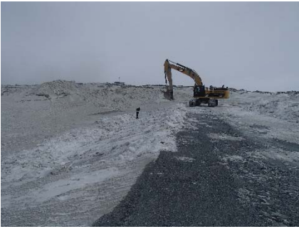
SD3-297 (2018-05-14), looking SE from Sta. 20+730/-10 m. Removal of snow on the upstream slope of SD3 with an excavator, from Sta. 20+640 to 20+760 m.
