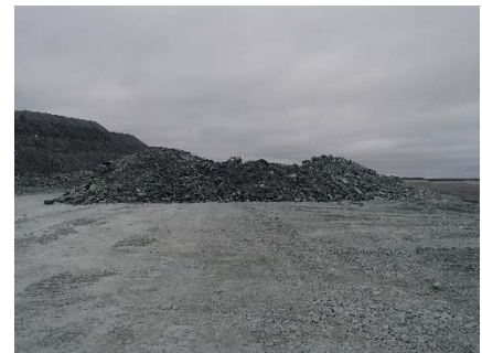
NCIS-090 (2018-07-13), looking SE from Sta. 2+440/-1 m (approx.). Placement of a 2 m thick (approx.) lift of UM rockfill from El. 152 m to El. 154 m (approx.) with a dozer from Sta. 2+455 m to 2+370 m (+4 m to -24 m).
