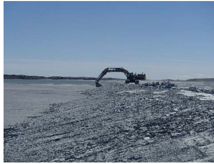
NCIS-056 (2018-06-28), looking S from Sta. 1+290/-39 m. Profiling of the upstream slope (3H:1V) from El. 148 to 150 m with an excavator from Sta. 1+340 m to 1+130 m.
