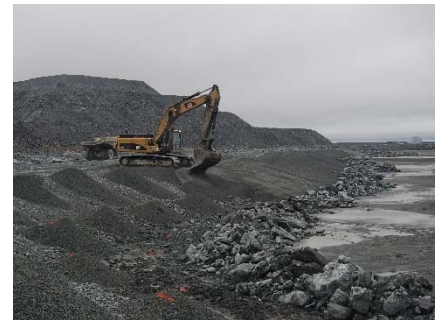
NCIS-042 (2018-06-25), looking SE from Sta. 2+210/-27 m. Placement of a 0.5 m thick lift of fine filter over the coarse filter in the upstream slope from El. 150 m to 152 m with an excavator from Sta. 2+305 m to 2+040 m.
