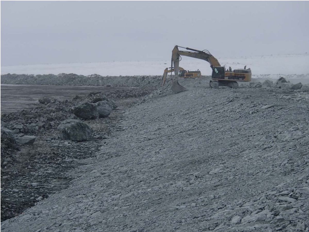
Photograph NCIS-007: Profiling of the upstream slope (3H:1V) from El. 150 to 152 m with an excavator.
