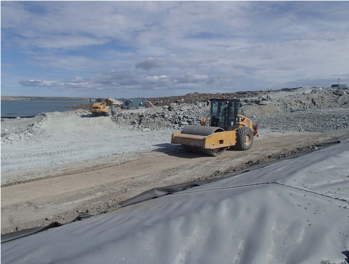
Photograph SD3-351: From Sta. 20+740/-24 m, looking SE. Compaction of the 0.5 m lift of low quality till (0-150 mm) at El. 143.5 m with a 10-tonne smooth-drum compactor with vibration (4 passes) from Sta. 20+619 m to 20+777 m.
