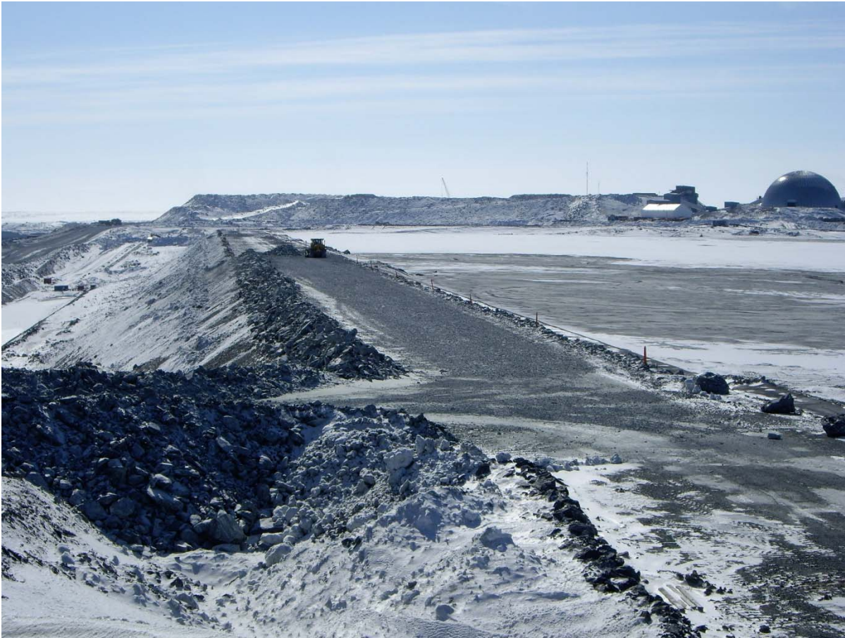
Photograph CD-1799: From Sta. 0+080/-25 m looking S. Placement a 2 m thick (approx.) lift of volcanic rockfill from El. 143 m to El. 145 m from 0+340 to 0+435 m (o.s. -28 to -18 m).
