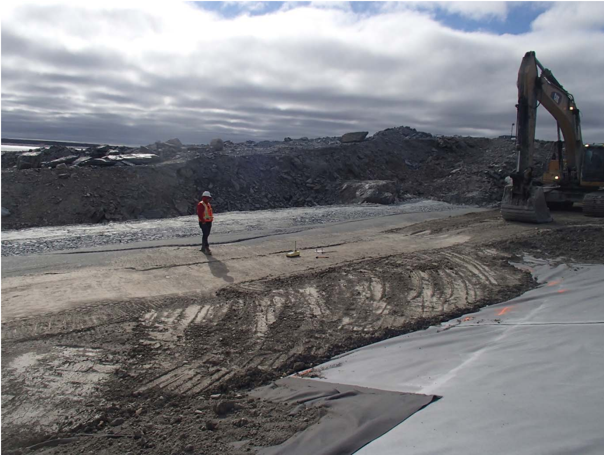
Photograph SD3-334: From Sta. 20+780/-26 m, looking SE. Compaction of the second 0.5 m thick lift of compacted sieved till and third lift of fine filter, coarse filter and fine rockfill of the upstream toe liner tie-in with a 10-tonne smooth-drum compactor with vibrations from Sta. 20+770 m to 20+800 m.
