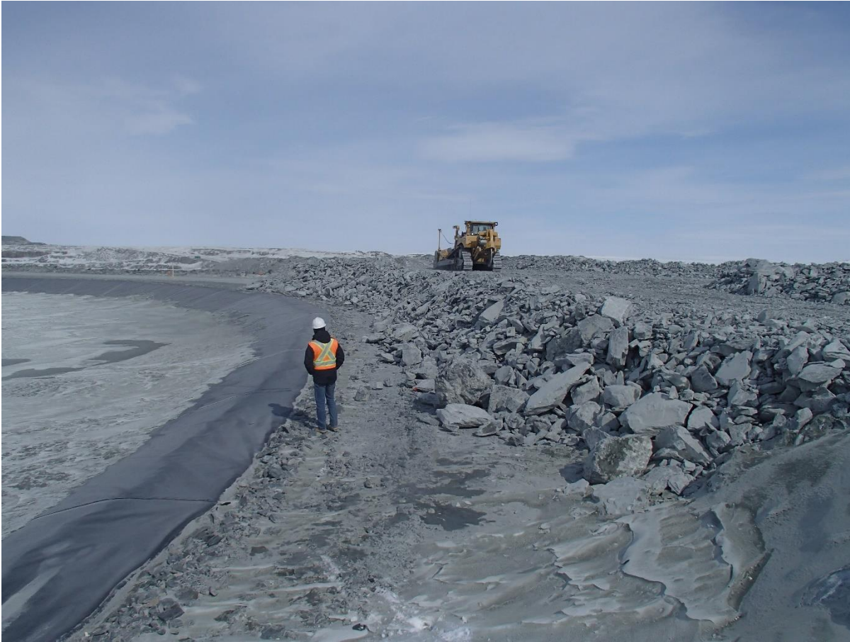
Photograph CD-1817: From Sta. 40+700/-10, looking NE. View of the rockfill lift thickness at the junction of Saddle Dam 5 and Central Dike, approx. 2.5 m thick.
