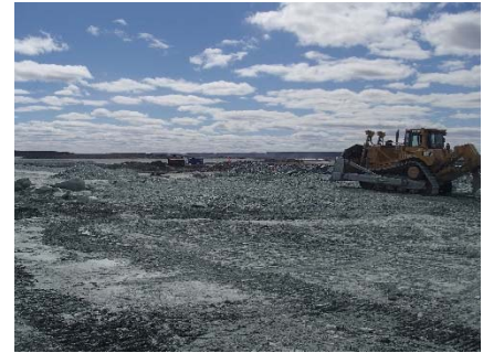
NCIS-060 (2018-06-29), looking SW from Sta. 1+365/-35 m. Placement of a 2 m thick (approx.) lift of UM rockfill from El. 150 m to El. 152 m (approx.) with a dozer from Sta. 1+340 m to 1+320 m (-19 m to +16 m). The material is of good quality and is well graded.
