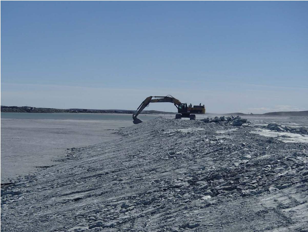
Photograph NCIS-056: From Sta. 1+290/-39 m (approx.), looking S. Profiling of the upstream slope (3H:1V) from El. 148 to 150 m with an excavator from Sta. 1+340 m to 1+130 m.
