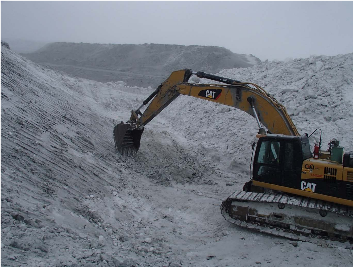
Photograph CD-1805: From Sta. 40+780/2 m looking NE. Final clean-up of footprint with an excavator to reach a good quality bedrock from Sta. 40+780 to 40+805 m (o.s. -6 to 9 m).
