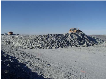
NCIS-091 (2018-07-14), looking S from Sta. 2+330/+13 m (approx.). Placement of a 2 m thick (approx.) lift of UM rockfill from El. 152 m to El. 154 m (approx.) with a dozer from Sta. 2+370 m to 2+290 m (+9 m to -22 m).
