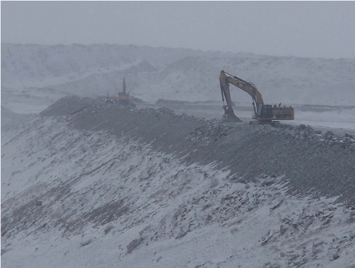
Photograph CD-1850: From Sta. 0+160/+20 m, looking SW. Profiling of the downstream slope (1.5H:1V) from El. 143 to 145 m with an excavator between Sta. 0+440 m and 0+530 m and between Sta. 0+745 m and 0+835 m.
