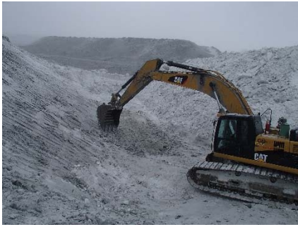
CD-1805 (2018-04-28), looking NE from Sta. 40+780/+2 m. Placement a 1.5 m thick (approx.) lift of intermediate volcanic (IV) rockfill from approx. Sta. 40+780 to 40+805 m (o.s. -6 to 9 m).
