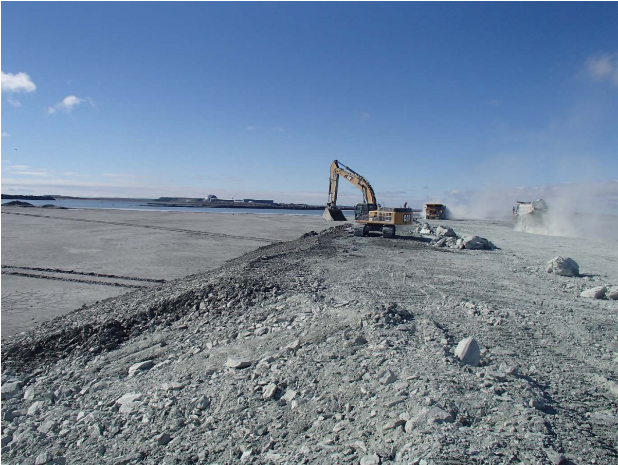
Photograph NCIS-058: From Sta. 1+340/-34 m (approx.), looking S. Placement of a 0.5 m thick lift of coarse filter in the upstream slope from El. 148 m to 152 m with an excavator from Sta. 1+340 m to 1+270 m.
