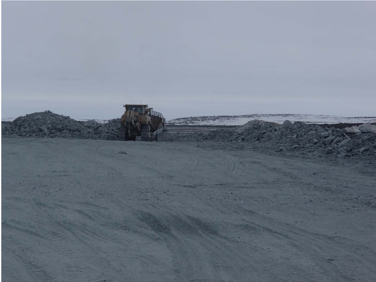
Photograph NCIS-021: From Sta. 1+550 m (approx.), looking S. Placement a 2 m thick (approx.) lift of UM rockfill from El. 150 m to El. 152 m (approx.) with a dozer from Sta. 1+535 m to 1+500 m (o.s. unavailable).
