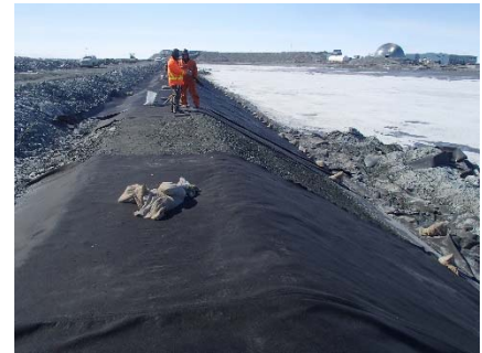
CD-1882 (2018-06-02), looking S from Sta. 0+510/-25 m. View of the emplacement of the geotextile panel with a horizontal weld in the slope at Sta. 0+520 following its removal.
