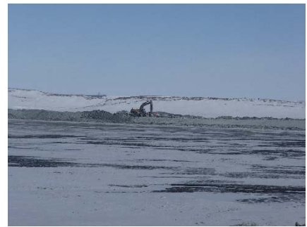
NCIS-018 (2018-05-25), looking NW from Sta. 2+310 m. Profiling of the upstream slope (3H:1V) from El. 150 to 152 m with an excavator from Sta. 1+989 m to 1+860 m.
