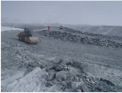
CD-1823 (2018-05-04), looking NE from Sta. 40+725/+8 m. Compaction of the two 2 m lifts (approx.) of intermediate volcanic (IV) rockfill at El. 143 and at El. 145 m with a 10-tonne smooth-drum compactor with vibration (6 passes) from Sta. 40+720 m to 40+750 m (o.s. -10 to +10 m).
