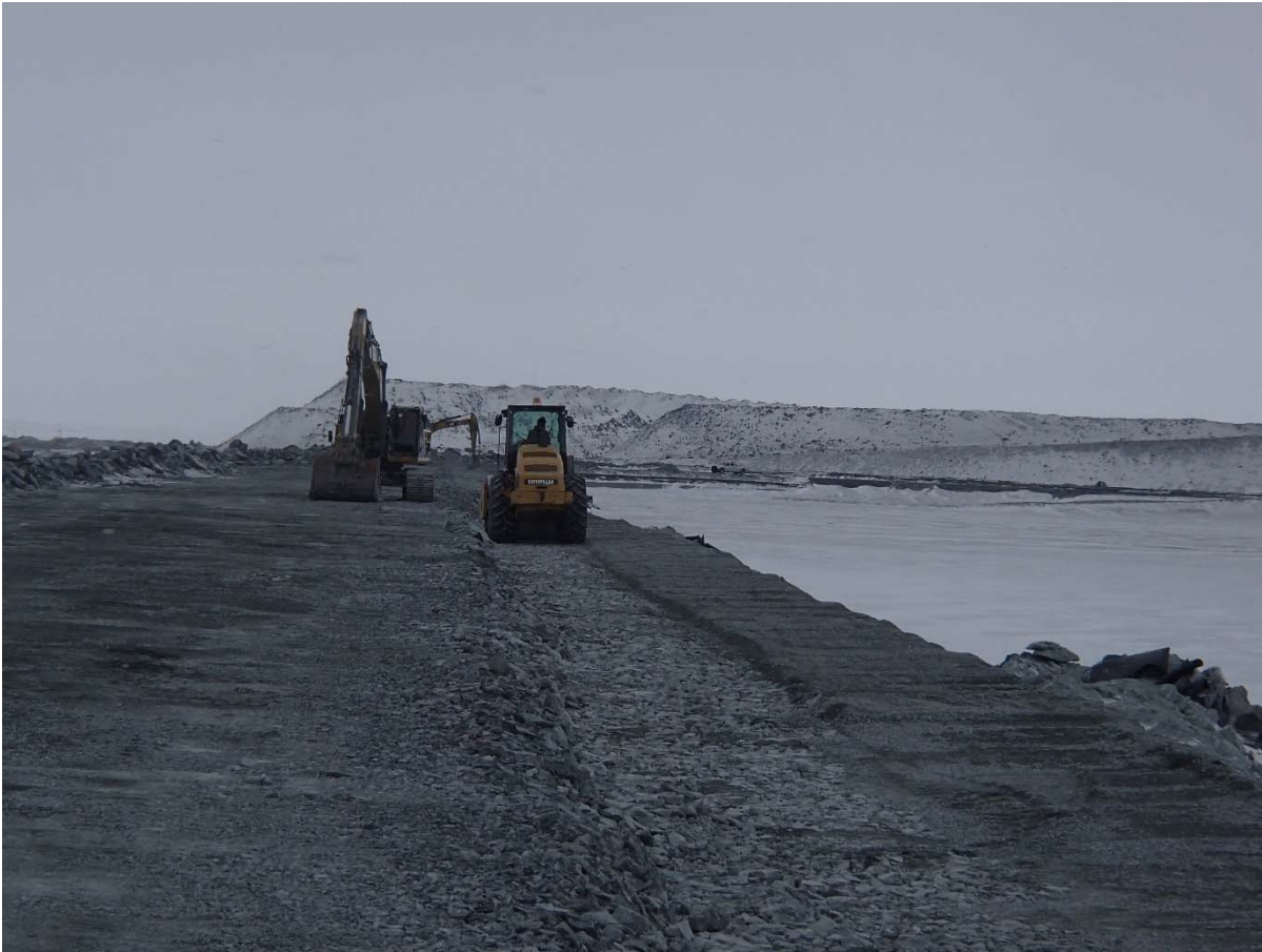
Photograph CD-1843: From Sta. 0+460/-23 m, looking S. Compaction of the third 0.5 m lift (approx.) of fine and coarse filters material at El. 144.5 m with a 10-tonne smooth-drum compactor with vibration (4 passes) from Sta 0+335m to 0+900 m.
