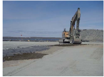
SD3-352 (2018-07-19), looking SW from Sta. 20+580/-49 m. View of SD3 at the end of the 2018 construction phase.
