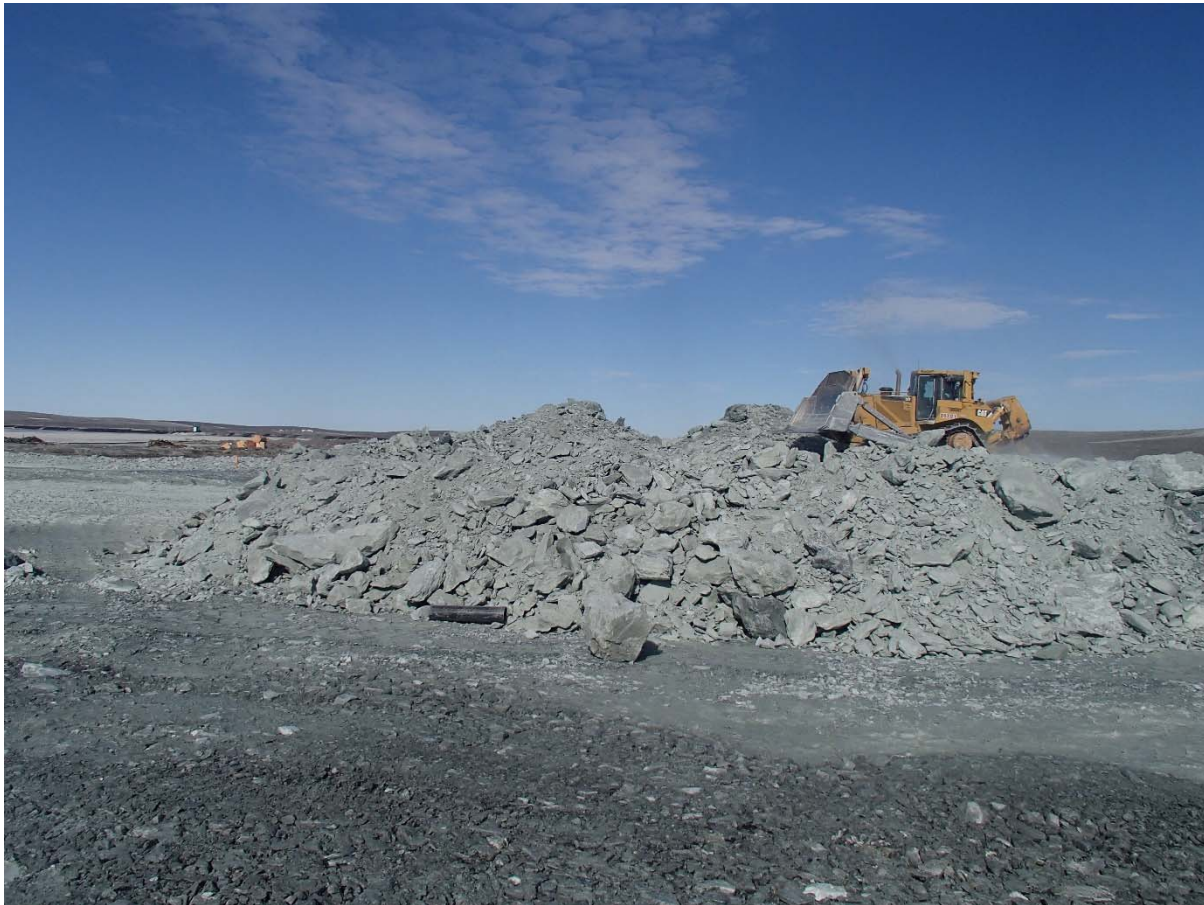
Photograph NCIS-064: From Sta. 1+200/-65 m (approx.), looking W. Placement of a 2 m thick (approx.) lift of UM rockfill from El. 150 m to El. 152 m (approx.) with a dozer from Sta. 1+320 m to 1+235 m (-65 m to -45 m). The material is of good quality and is well graded.
