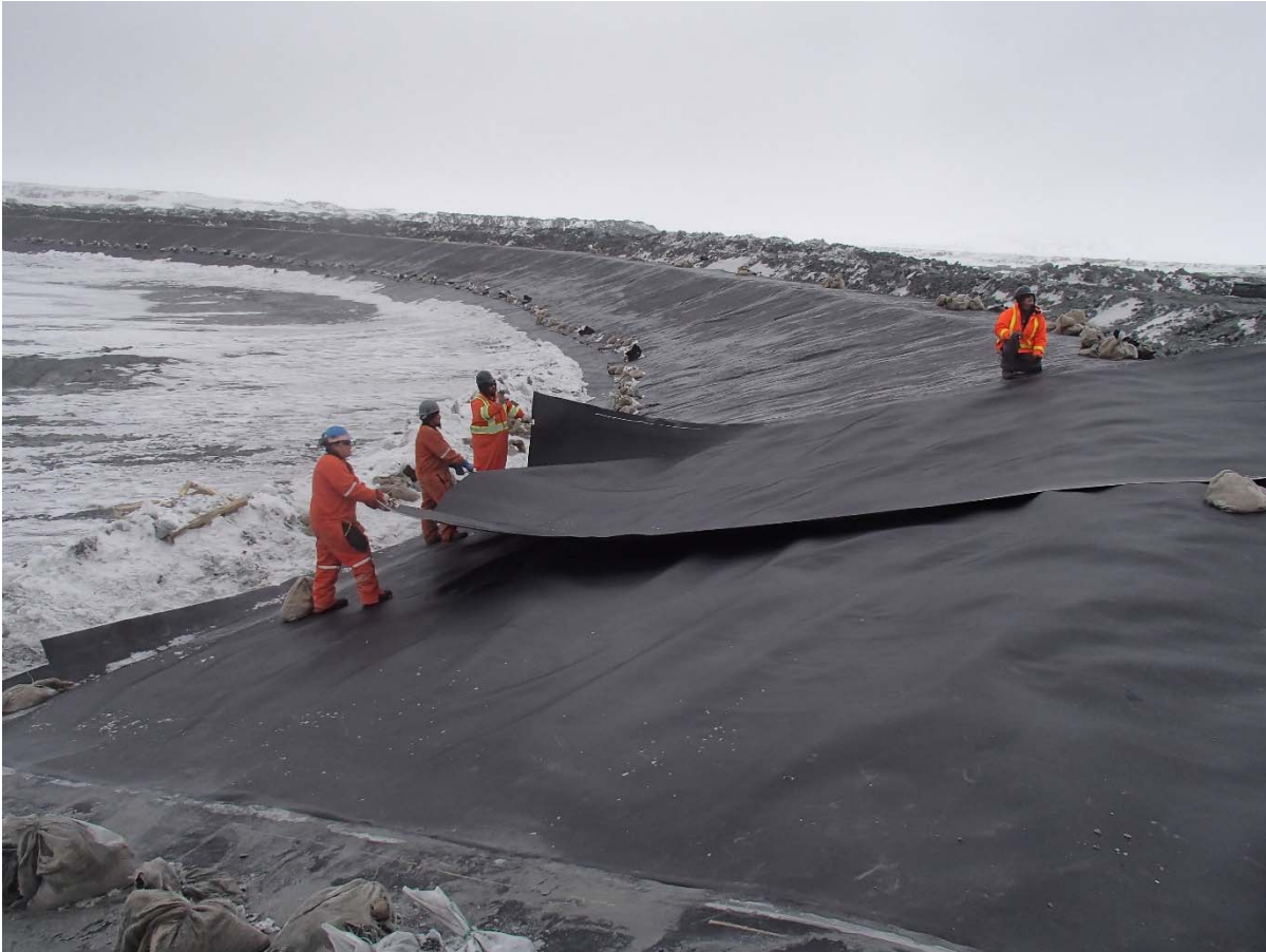
Photograph CD-1861: From Sta. 40+680/-28 m, looking NE. Installation of the LLDPE liner on the upstream slope 3H:1V (SD5 side) to 2H:1V (Central Dike side) between El. 143 m and 145 m from Sta. 40+680 m to 0+950 m (panel numbers 802 to 817).
