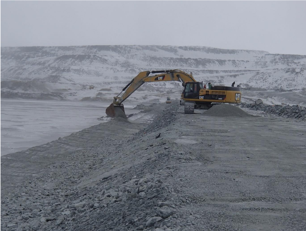
Photograph CD-1836: From Sta 0+830/-20m, looking N. Placement of a first 0.5 m thick lift of fine filter from El. 143 m to 143.5 m upstream of the coarse filter with an excavator from Sta. 0+490 to 0+835 m.
