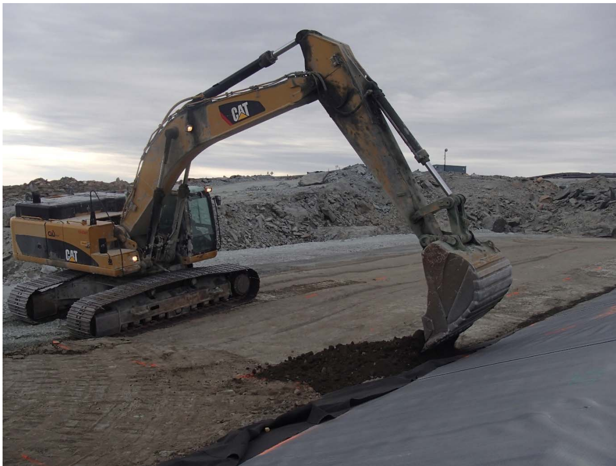
Photograph SD3-348: From Sta. 20+760/-25 m, looking E. Placement of a 0.5 m thick layer of compacted sieved till on the upstream slope of SD3 with an excavator from Sta. 20+777 m to 20+807 m. No large rock was allowed to be placed against the LLDPE liner.
