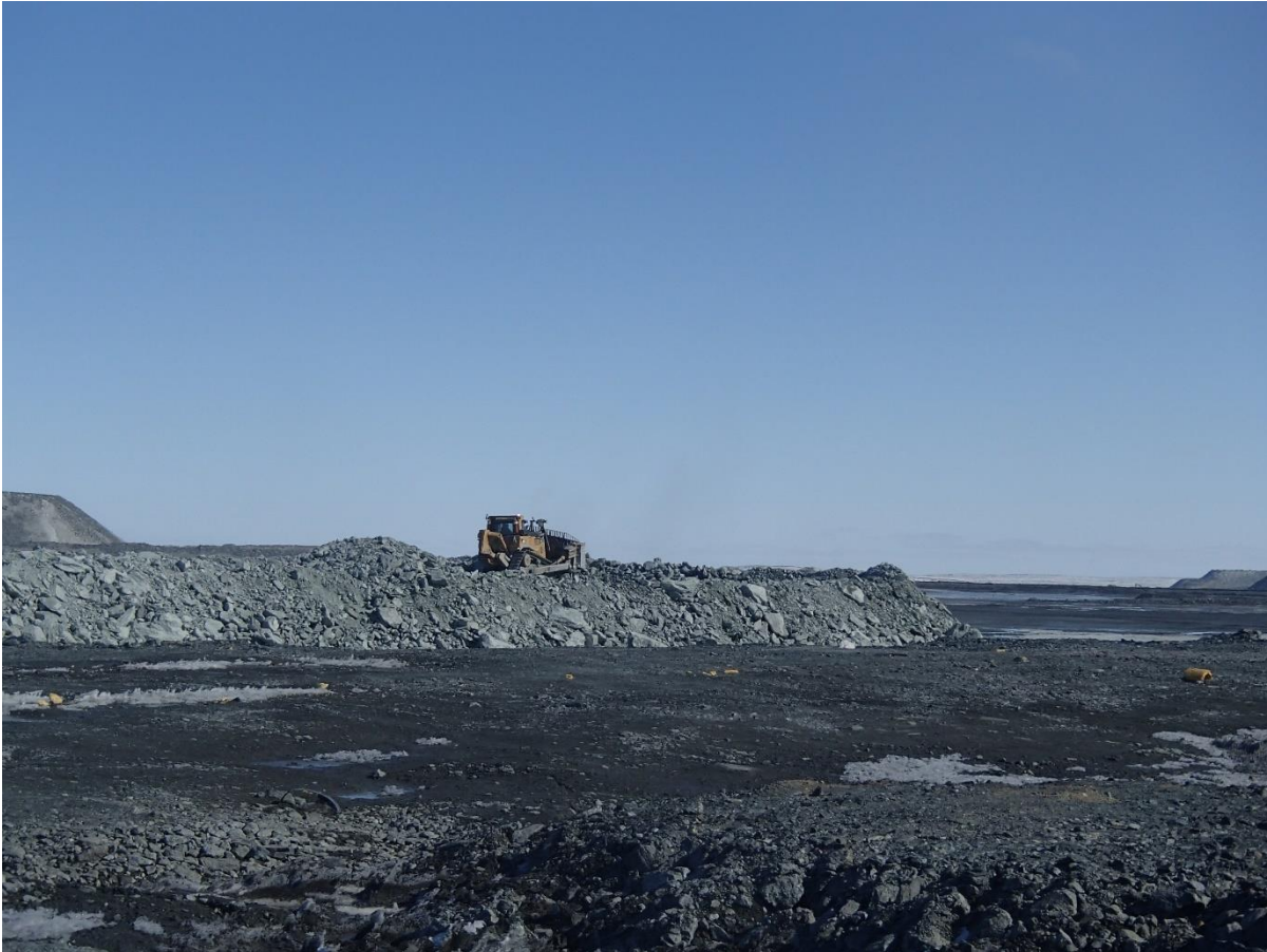
Photograph NCIS-025: From Sta. 1+475 m (approx.), looking SE. Placement of a 2 m thick (approx.) lift of UM rockfill from El. 150 m to El. 152 m (approx.) with a dozer from Sta. 1+450 m to 1+390 m (o.s. unavailable). The material is of good quality and is well graded.
