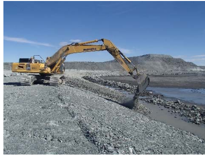
NCIS-029 (2018-06-19), looking SE from Sta. 2+120/-27 m. Placement of a 0.5 m thick lift of coarse filter in the upstream slope from El. 150 m to 152 m with an excavator from Sta. 2+280 m to 2+105 m.
