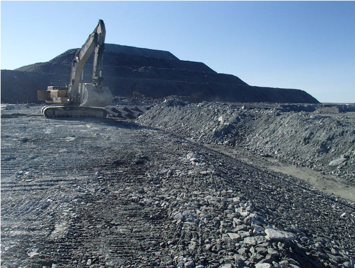
Photograph NCIS-051: From Sta. 2+630/-34 m (approx.), looking SE. Placement of a 0.5 m thick lift of coarse filter in the upstream slope from El. 150 m to 152 m with an excavator from Sta. 2+640 m to 2+815 m.
