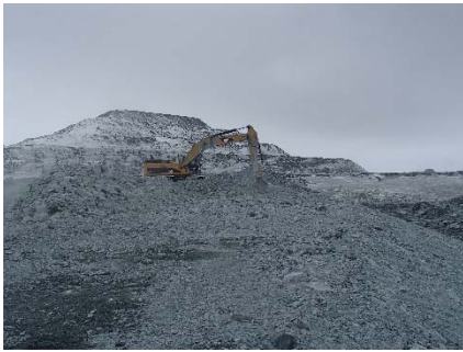
NCIS-013 (2018-05-22), looking NE from Sta. 2+600 m. Correction of the crest elevation with an excavator to achieve a closer elevation to 152 m around Sta. 2+650 m.
