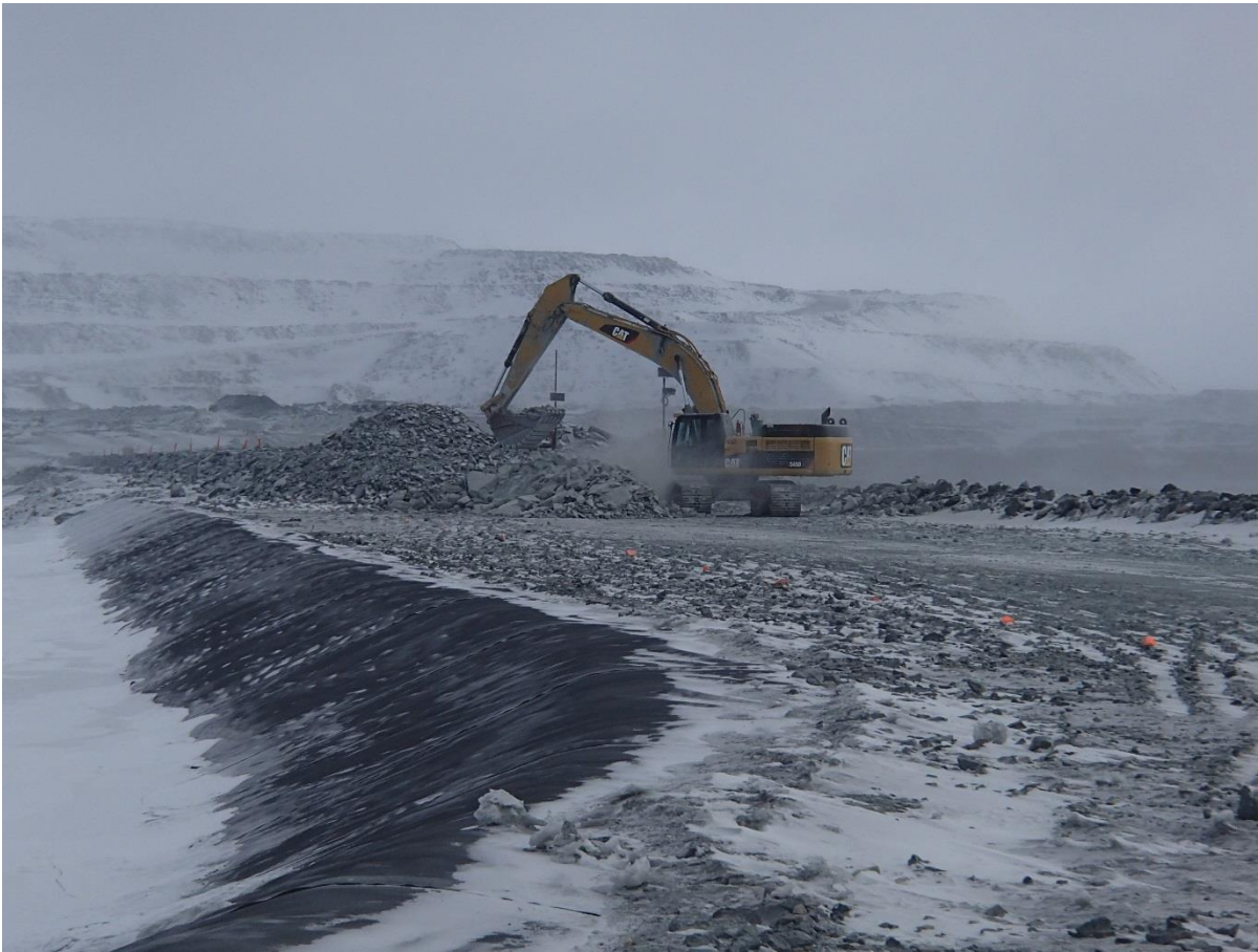
Photograph CD-1814: From Sta. 0+970/-10, looking NE. Placement of intermediate volcanic (IV) rockfill around the instruments at approx. Sta. 0+830 m with the excavator.
