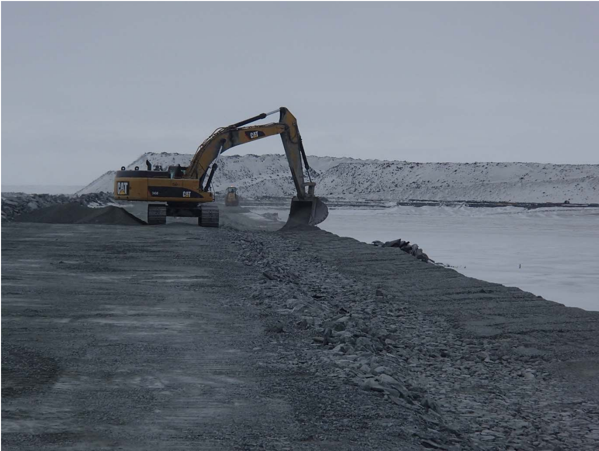
Photograph CD-1842: From Sta. 0+380/-16 m, looking S. Placement of a third 0.5 m thick lift of fine filter from El. 143.5 m to 144 m upstream of the coarse filter with an excavator from Sta. 0+335 m to 0+940 m.
