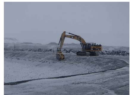
CD-1849 (2018-05-13), looking NE from Sta. 40+750/-17 m. Final rolling of the upstream slope in view of the LLDPE geomembrane installation from Sta. 0+170 m to 40+730 m.
