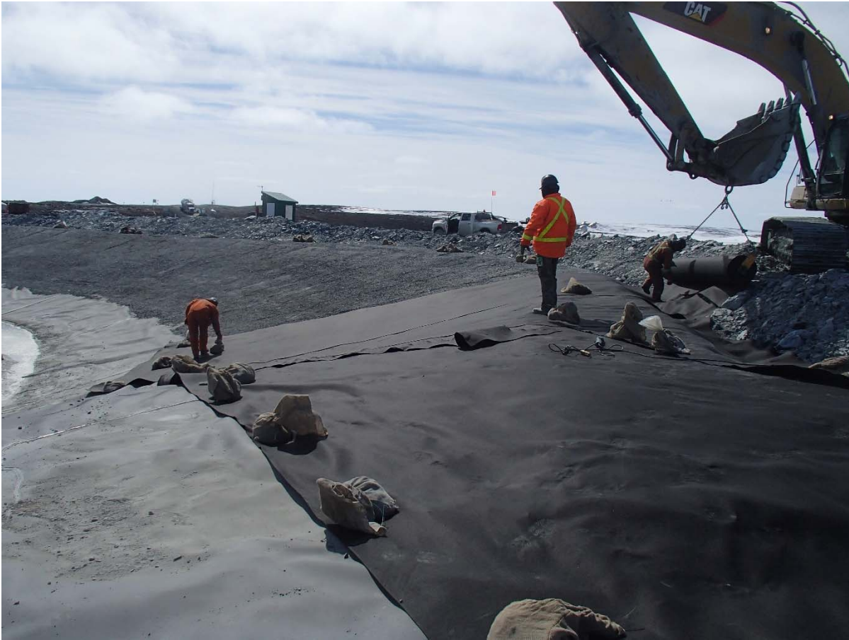
Photograph SD3-308: From Sta. 20+620/-48 m, looking SW. Installation of the geotextile on the upstream slope 3H:1V between El. 143 m and 145 m from Sta. 20+610 m to 20+810 m.
