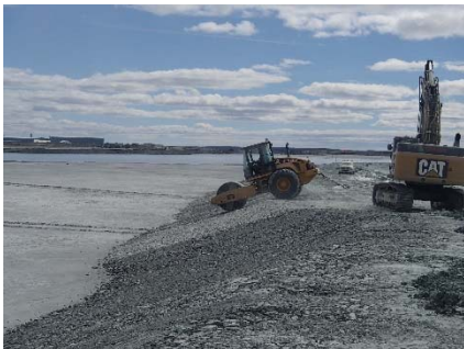
NCIS-061 (2018-06-29), looking S from Sta. 1+365/-35 m. Compaction of the 0.5 m lift of coarse filter between El. 148 and 152 m with a 10-tonne smooth-drum compactor with vibration (4 passes) in the upstream slope from Sta. 1+340 m to 1+270 m.
