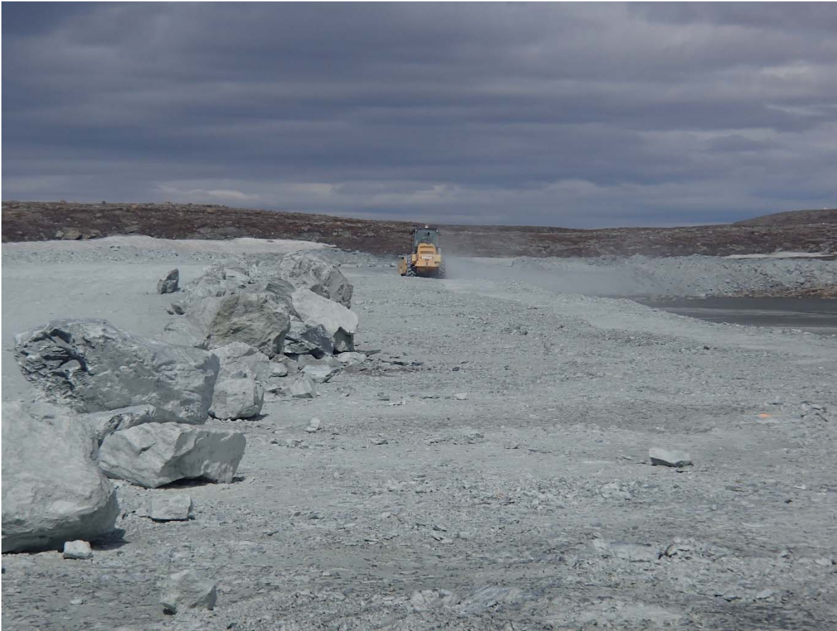
Photograph NCIS-032: From Sta. 1+400/-24 m (approx.), looking N. Compaction of the 2 m lift (approx.) of ultramafic (UM) rockfill at El. 152 m with a 10-tonne smooth-drum compactor with vibration (6 passes) between the haul truck traffic lane and the upstream slope from Sta. 1+660 to 1+380 m (o.s. -45 to -24 m).
