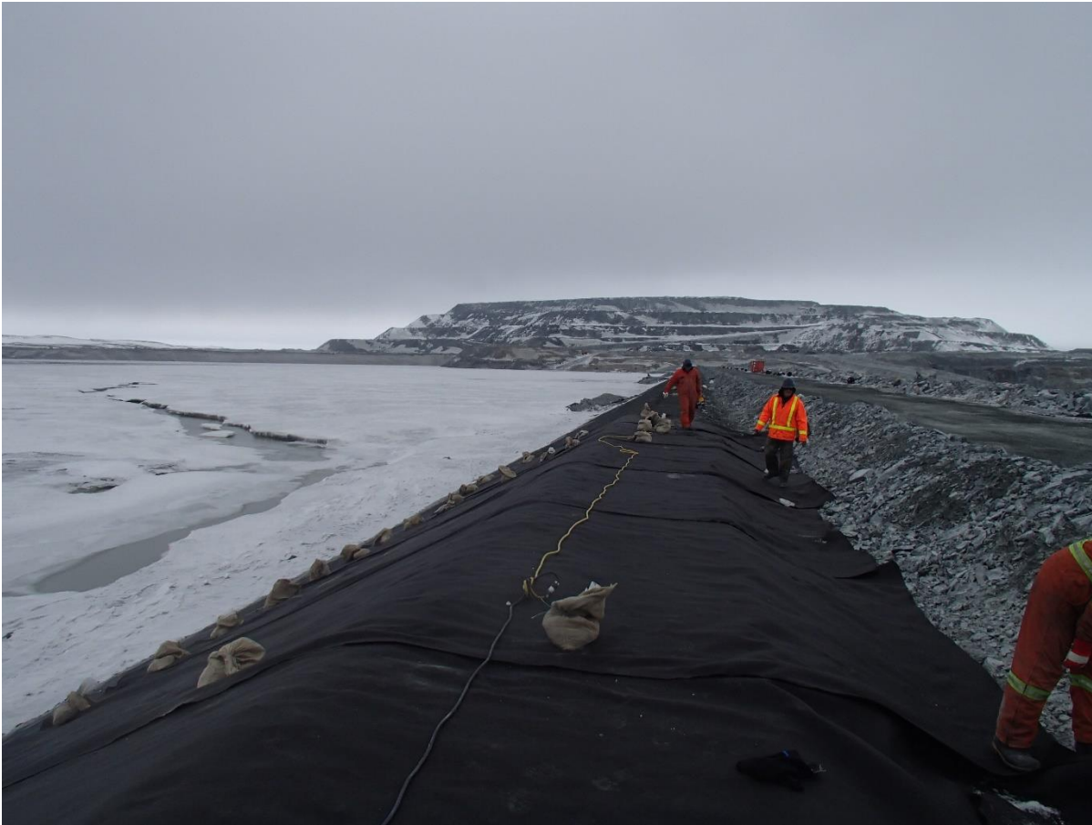
Photograph CD-1873: From Sta. 0+760/-26 m, looking N. Installation of the geotextile on the upstream slope 2H:1V between El. 143 m and 145 m from Sta. 0+760 m to 0+740 m.
