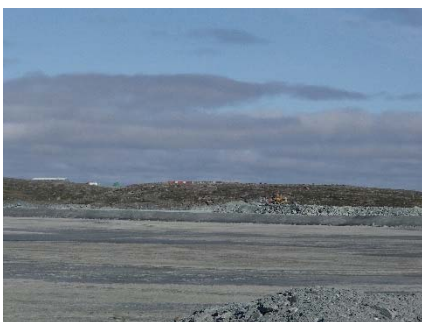
NCIS-106 (2018-07-21), looking NW from Sta. 2+620/-35 m (approx.). Placement of a 2 m thick (approx.) lift of UM rockfill from El. 152 m to El. 154 m (approx.) with a dozer from Sta. 1+947 m to 1+863 m (+14 m to -26 m).
