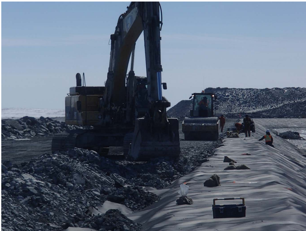
Photograph CD-1884: From Sta. 0+530/-25 m, looking S. Backfilling of the geosynthetics tie-in from Sta. 0+610 m to 0+480 m and compaction of the tie-in material with a 10-tonne smooth-drum compactor with vibration (4 passes) from Sta. 0+610 to 0+480 m.
