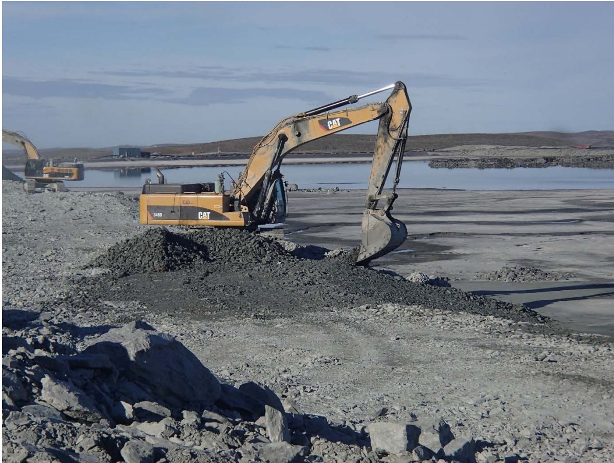
Photograph NCIS-076: From Sta. 2+940/-15 m (approx.), looking SW. Placement of a 0.5 m thick lift of coarse filter in the upstream slope from El. 150 m to 152 m with an excavator from Sta. 2+980 m to 3+160 m.
