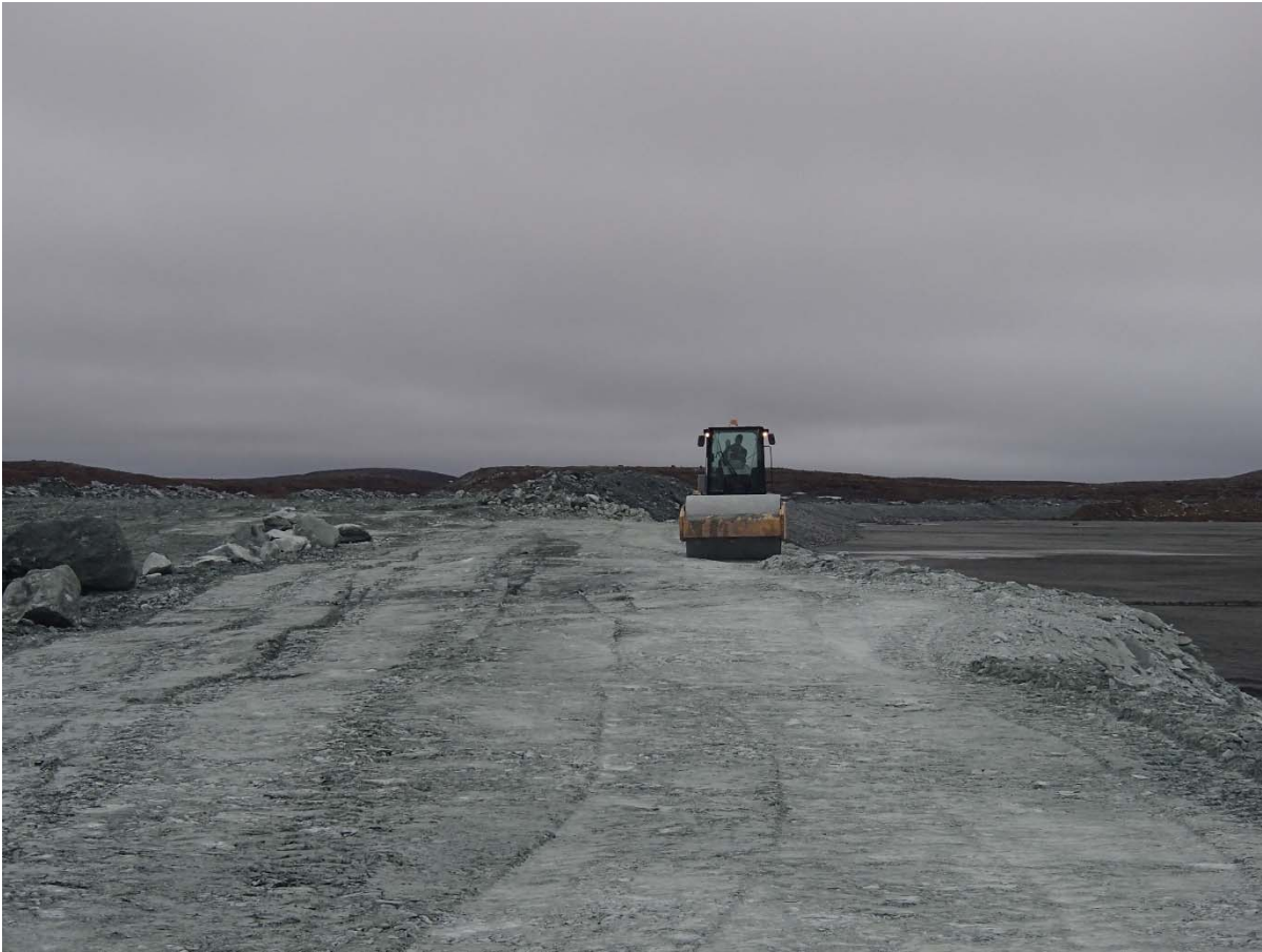
Photograph NCIS-043: From Sta. 1+250/-38 m (approx.), looking N. Compaction of the 1.5 to 2 m lift (approx.) of ultramafic (UM) rockfill at El. 150 m with a 10-tonne smooth-drum compactor with vibration (6 passes) between the haul truck traffic lane and the upstream slope from Sta. 1+330 to 1+200 m (offset -53 to -24 m).
