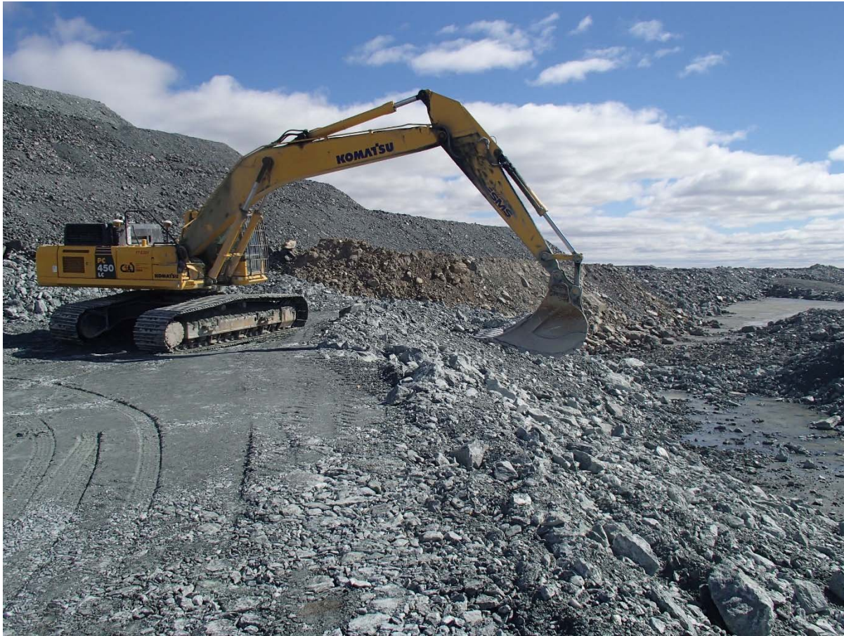
Photograph NCIS-045: From Sta. 2+760/-40 m (approx.), looking S. Profiling of the upstream slope (3H:1V) from El. 150 to 152 m with an excavator from Sta. 2+715 m to 2+825 m.
