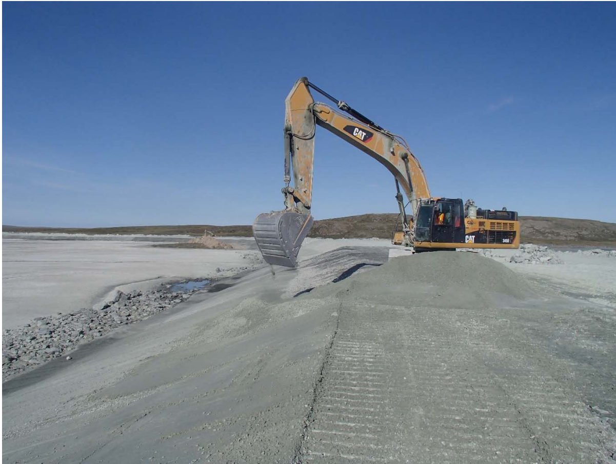
Photograph NCIS-117: From Sta. 2+050/-25 m (approx.), looking SW. Placement of a 0.5 m thick lift of fine filter in the upstream slope from El. 152 m to 154 m with an excavator from Sta. 2+090 m to 1+890 m.
