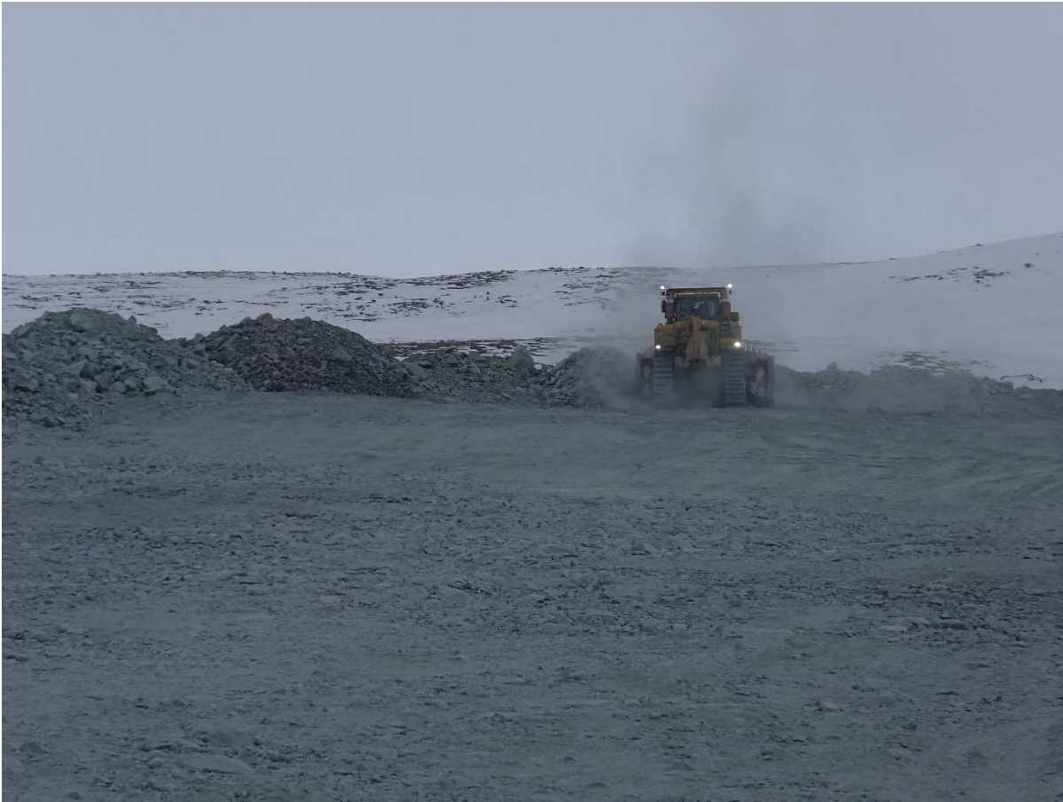
Photograph NCIS-011: From Sta. 2+000 m (approx.), looking SW. Placement a 2 m thick (approx.) lift of UM rockfill from El. 150 m to El. 152 m (approx.) with a dozer from Sta. 1+880 m to 1+767 m (offset unavailable).
