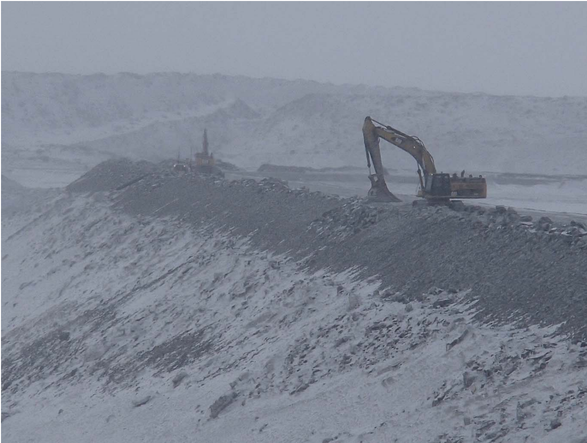
Photograph CD-1850: From Sta. 0+160/+20 m, looking SW. Profiling of the downstream slope (1.5H:1V) from El. 143 to 145 m with an excavator between Sta. 0+440 m and 0+530 m and between Sta. 0+745 m and 0+835 m.
