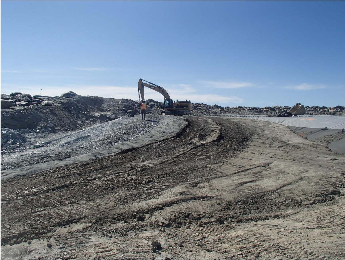
Photograph SD3-336: From Sta. 20+755/-48 m, looking S. Placement of a fourth 0.5 m thick lifts of fine filter, coarse filter and fine rockfill on the upstream slope of the upstream toe liner tie-in with an excavator from Sta. 20+770 to 20+800 m.
