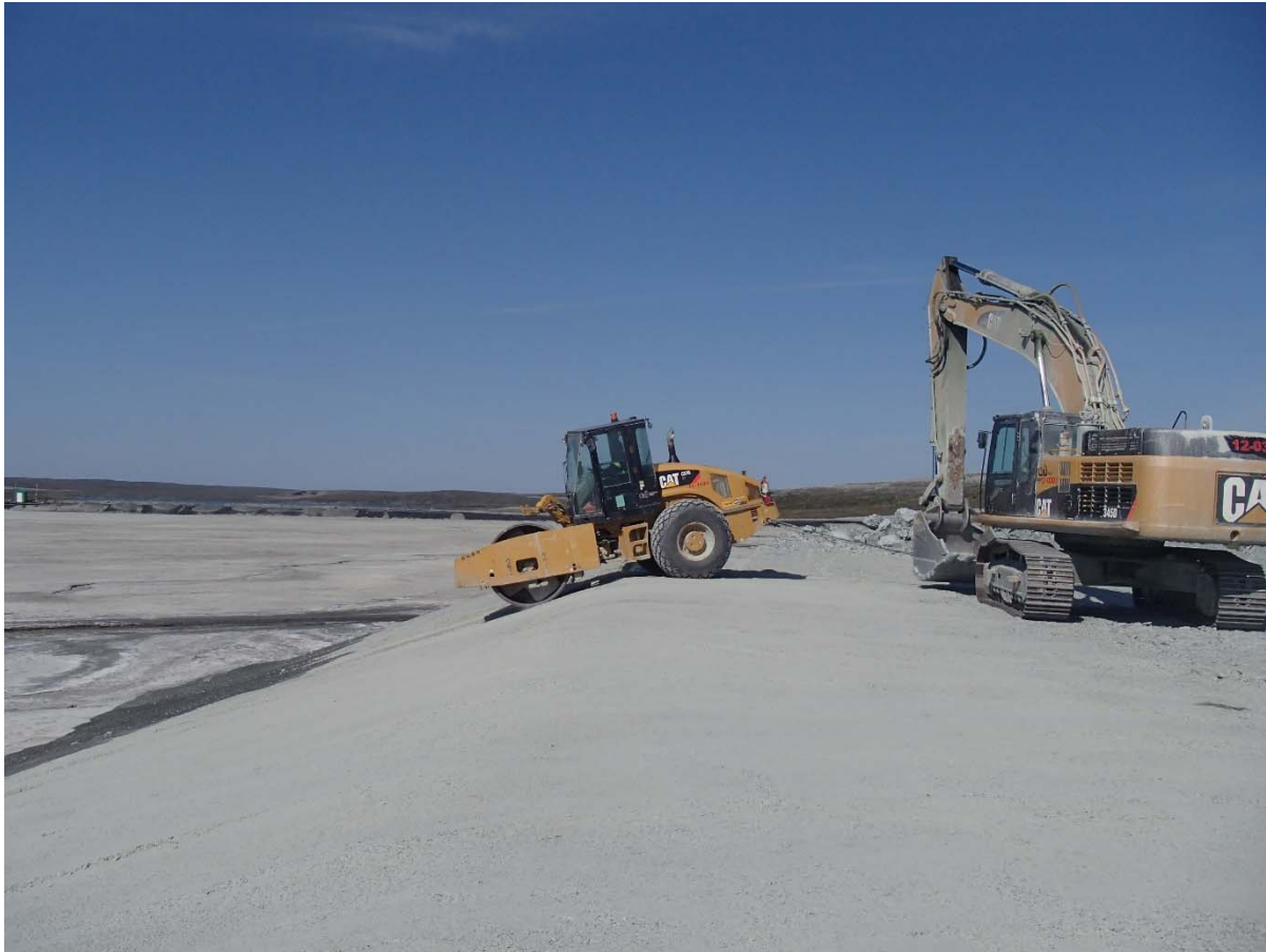
Photograph NCIS-126: From Sta. 1+140/-98 m (approx.), looking W. Compaction of the 0.5 m lift (approx.) of fine filter between El. 150 m and 152 m with a 10-tonne smooth-drum compactor with vibration (4 passes) in the upstream slope from Sta. 1+240 m to 1+100 m.
