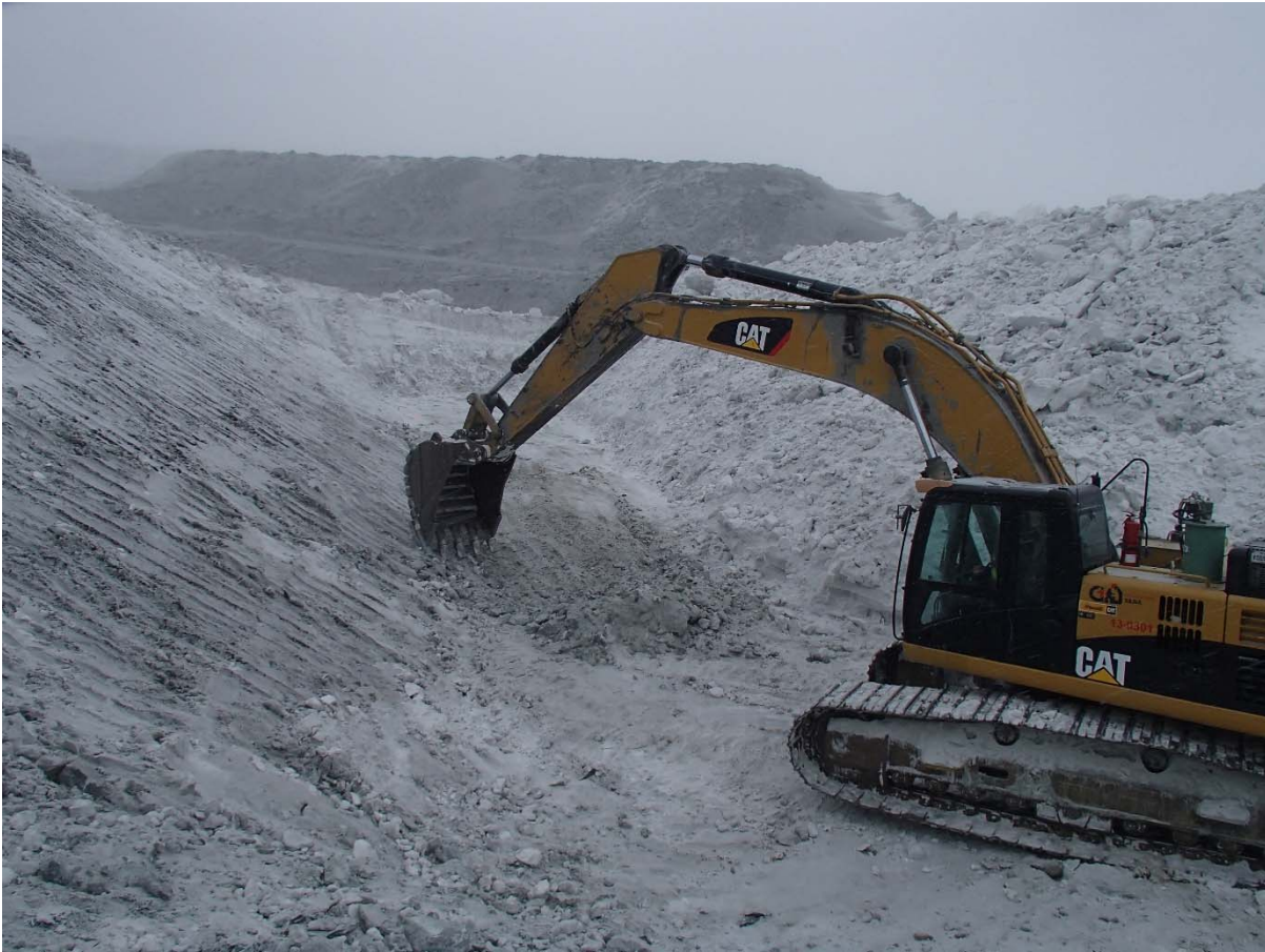
Photograph CD-1805: From Sta. 40+780/2 m looking NE. Final clean-up of footprint with an excavator to reach a good quality bedrock from Sta. 40+780 to 40+805 m (o.s. -6 to 9 m).
