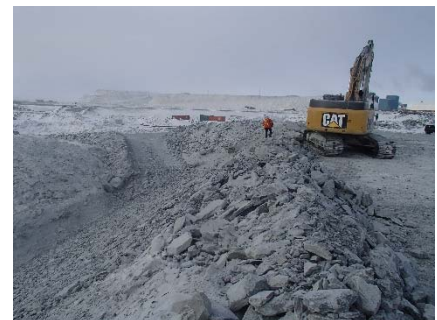
CD-1813 (2018-05-01), looking S from Sta. 0+980/-2 m. Placement of intermediate volcanic (IV) rockfill on the existing downstream slope up to approx. El. 143 m, from approx. Sta. 0+980 to 40+780 m.
