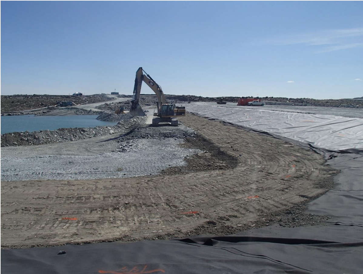
Photograph SD3-330: From Sta. 20+610/-43 m, looking S. Placement of a second 0.5 m thick lift of fine rockfill (0-500 mm) upstream of the low quality till (0-150mm) from El. 142.5 m to 143 m from Sta. 20+610 m to 20+760 m.
