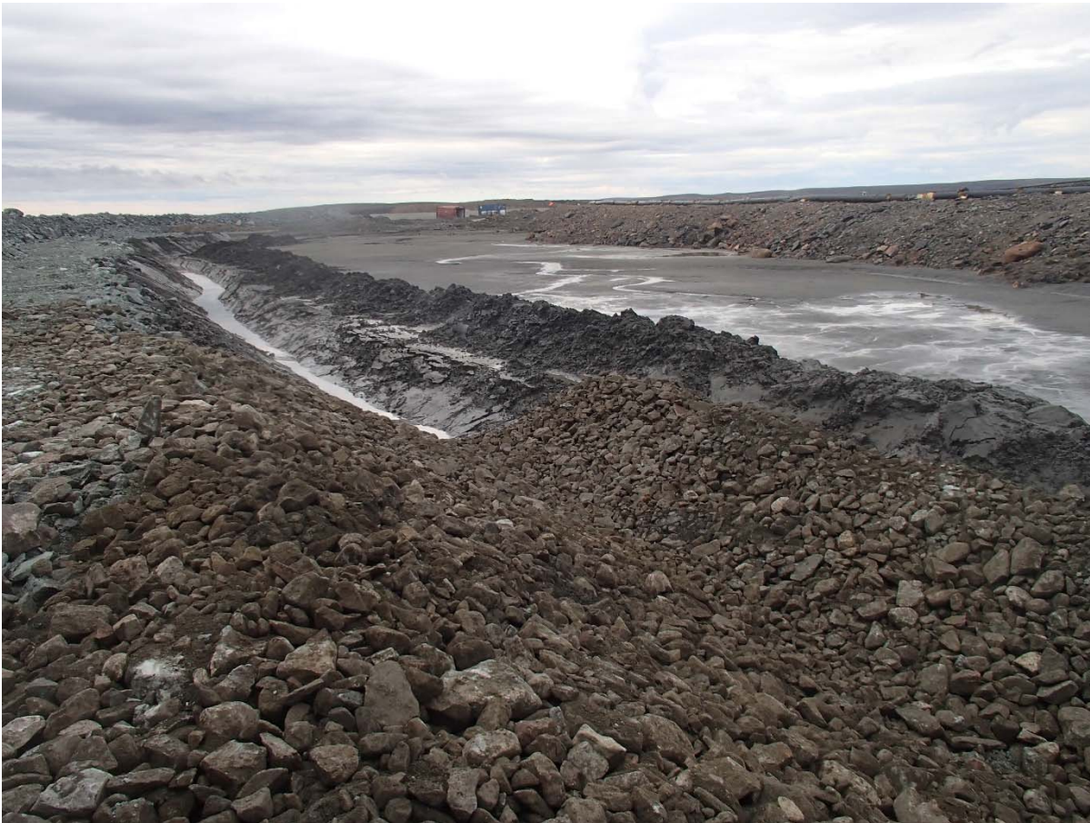
Photograph NCIS-138: From Sta. 1+365/+15 m (approx.), looking SW. Excavation of a 0.8 m (approx.) deep, 1 m wide shallow ditch in the tailings and placement of a 0.3 m thick (approx.) layer of till sieving reject material on the bottom and on the slopes of the ditch from Sta. 1+200 m to 1+100 m.
