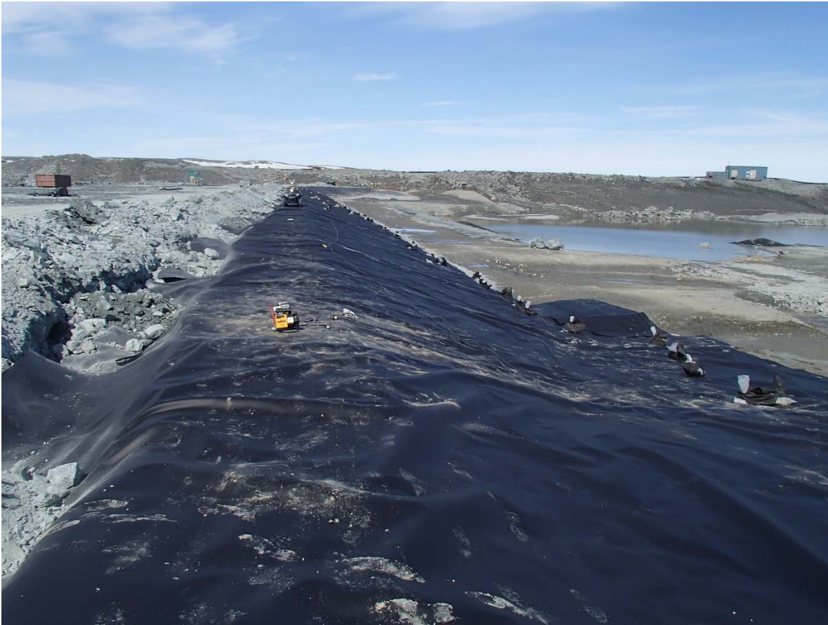
Photograph SD3-311: From Sta. 20+810/-26 m, looking N. Installation of the LLDPE liner on the upstream slope 3H:1V between El. 143 m and 145 m from Sta. 20+630 m to 20+800 m (panel numbers 939 to 964).
