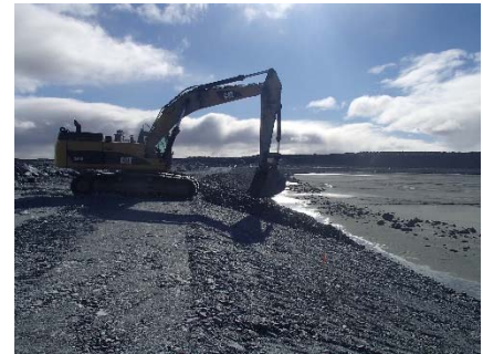
NCIS-033 (2018-06-21), looking E from Sta. 1+900/-21 m. Placement of a 0.5 m thick lift of coarse filter in the upstream slope from El. 150 m to 152 m with an excavator from Sta. 1+930 m to 1+715 m.
