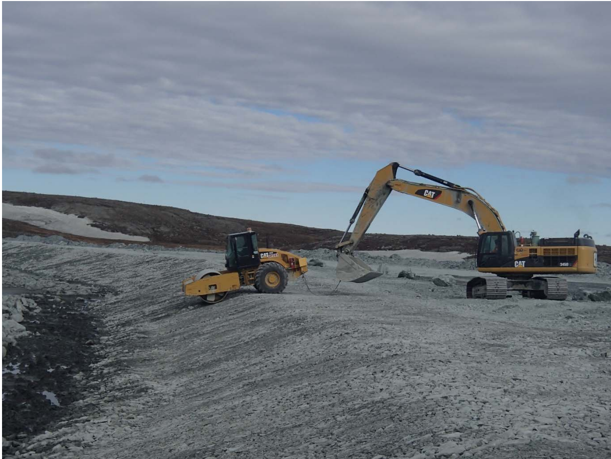
Photograph NCIS-037: From Sta. 1+550/-25 m (approx.), looking NW. Compaction of the 0.5 m lift (approx.) of coarse filter between El. 150 and 152 m with a 10-tonne smooth-drum compactor (4 passes) in the upstream slope from Sta. 2+450 to 1+805 m.
