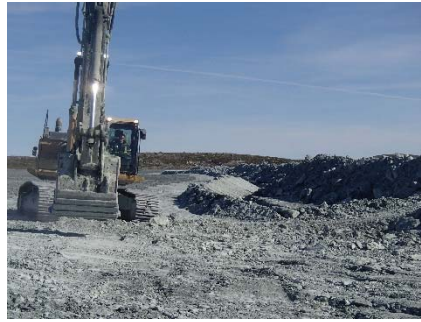
NCIS-119 (2018-07-26), looking N from Sta. 1+430/-22 m (approx.). Excavation of a 0.8 m (approx.) deep, 1 m wide shallow ditch in the rockfill capping with an excavator from Sta. 1+455 m to 1+400 m.
