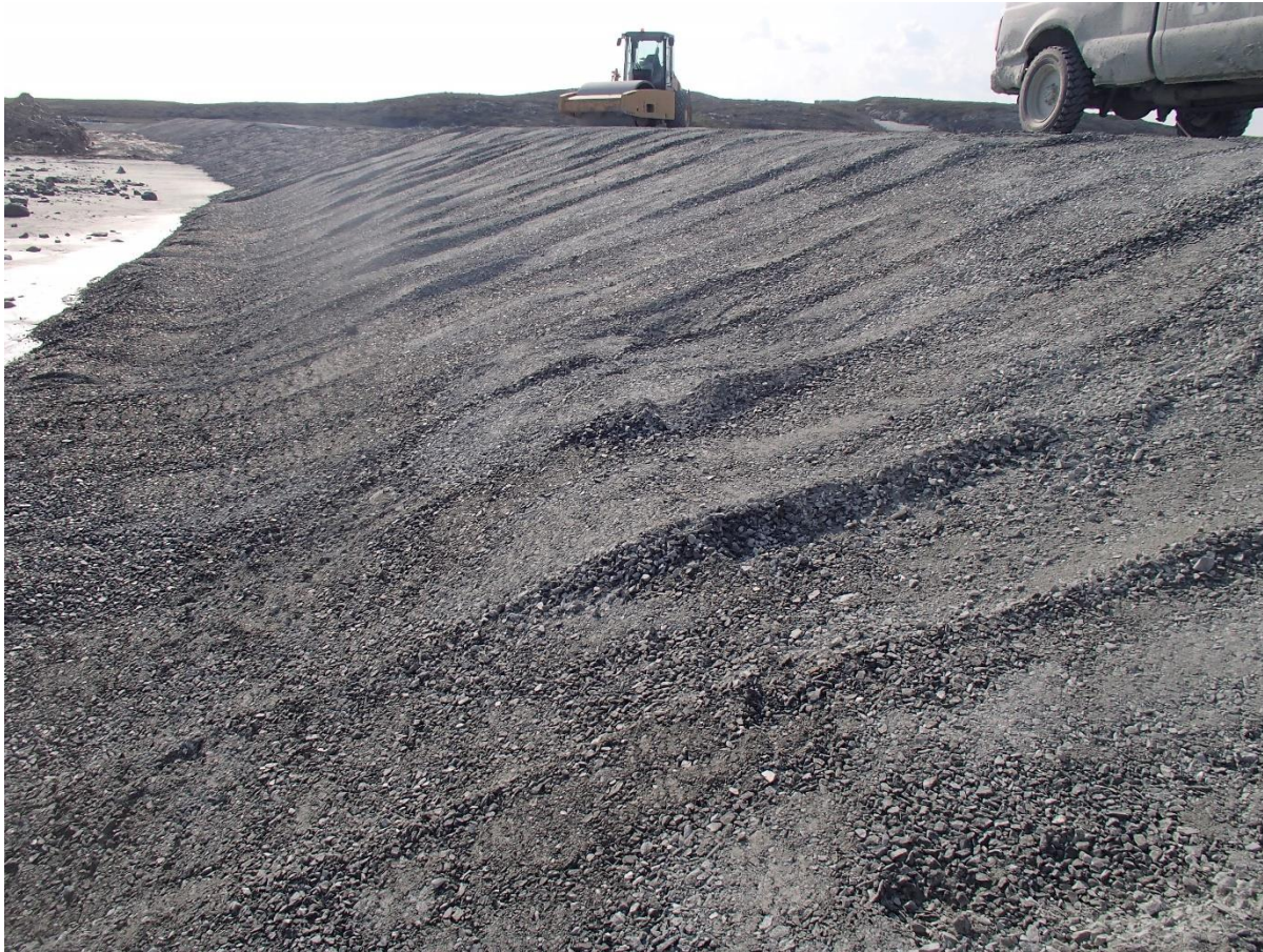
Photograph NCIS-087: From Sta 1+950/-34 m (approx.), looking W. Compaction of the 0.5 m lift (approx.) of fine filter between El. 150 and 152 m with a 10-tonne smooth-drum compactor (4 passes) in the upstream slope from Sta. 2+000 m to 1+930 m. Vibration is used except for the first pass down the slope in order to stabilize the material and limit deformation of the lift.
