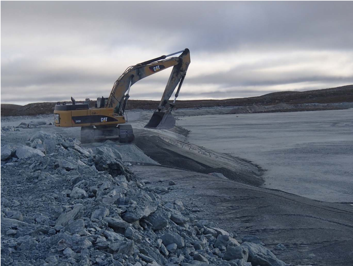
Photograph NCIS-073: From Sta. 1+300/-33 m (approx.), looking N. Placement of a 0.5 m thick lift of fine filter over the coarse filter in the upstream slope from El. 150 m to 152 m with an excavator from Sta. 1+320 m to 1+300 m.
