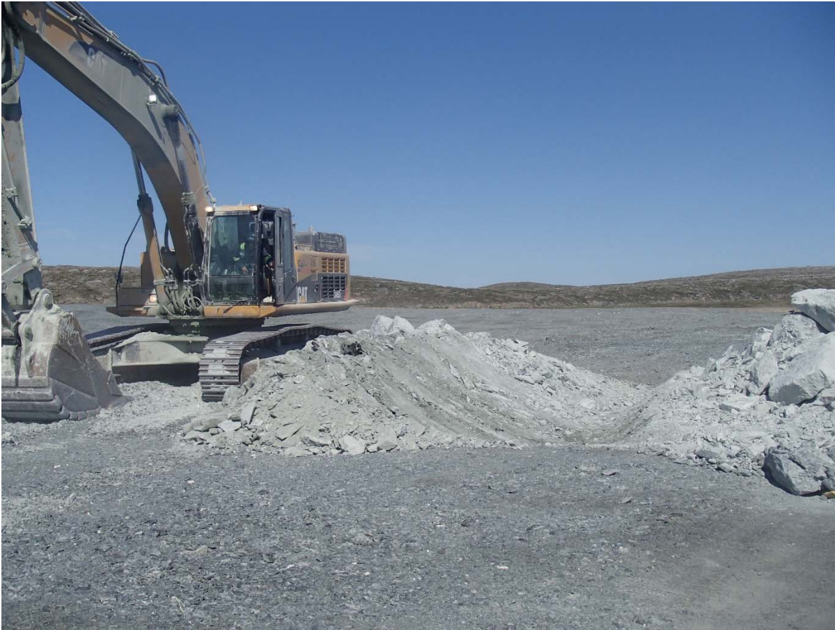
Photograph NCIS-114: From Sta. 1+700/-34 m (approx.), looking N. Excavation of a 0.8 m (approx.) deep, 1 m wide shallow ditch in the rockfill capping with an excavator from Sta. 1+500 m to 1+650 m.
