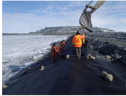
CD-1878 (2018-06-01), looking N from Sta. 0+720/-22 m. Installation of the LLDPE liner on the upstream slope 2H:1V between El. 143 m and 145 m from Sta. 0+740 m to 0+610 m (panel numbers 849 to 867).
