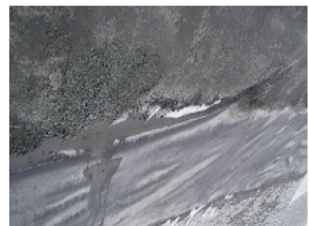
CD-1858 (2018-05-21), looking S from Sta. 0+970/-45 m. View of the bottom of the fine filter upstream slope. Some material is missing to achieve a smooth slope.
