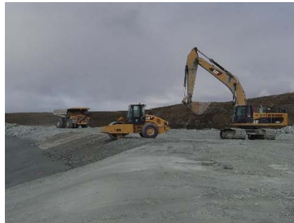
NCIS-131 (2018-07-29), looking W from Sta. 1+940/-20 m (approx.). Compaction of the 0.5 m lift (approx.) of coarse filter between El. 152 m and 154 m with a 10-tonne smooth-drum compactor with vibration (4 passes) in the upstream slope from Sta. 1+890 m to 1+826 m.
