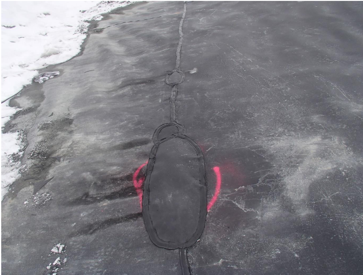
Photograph CD-1876: From Sta. 0+820/-26 m, looking N. View of repair patches on the extrusion weld at the bottom of panel 838.
