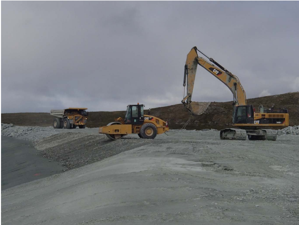
Photograph NCIS-131: From Sta. 1+940/-20 m (approx.), looking W. Compaction of the 0.5 m lift (approx.) of coarse filter between El. 152 m and 154 m with a 10-tonne smooth-drum compactor with vibration (4 passes) in the upstream slope from Sta. 1+890 m to 1+826 m.
