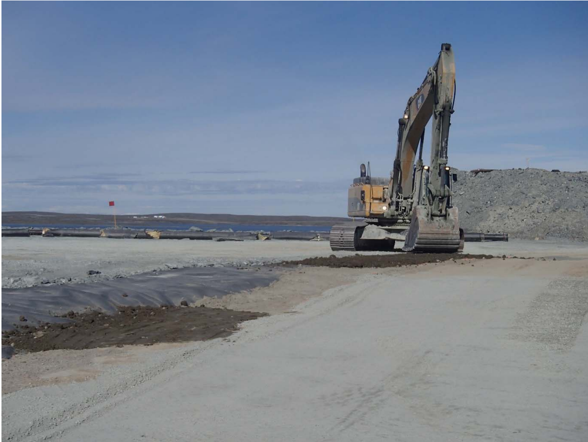
Photograph SD3-352: From Sta. 20+600/-59 m, looking SW. Corrections to the layer of compacted sieved till placed against the upstream slope from Sta. 20+599 m to 20+613 m.
