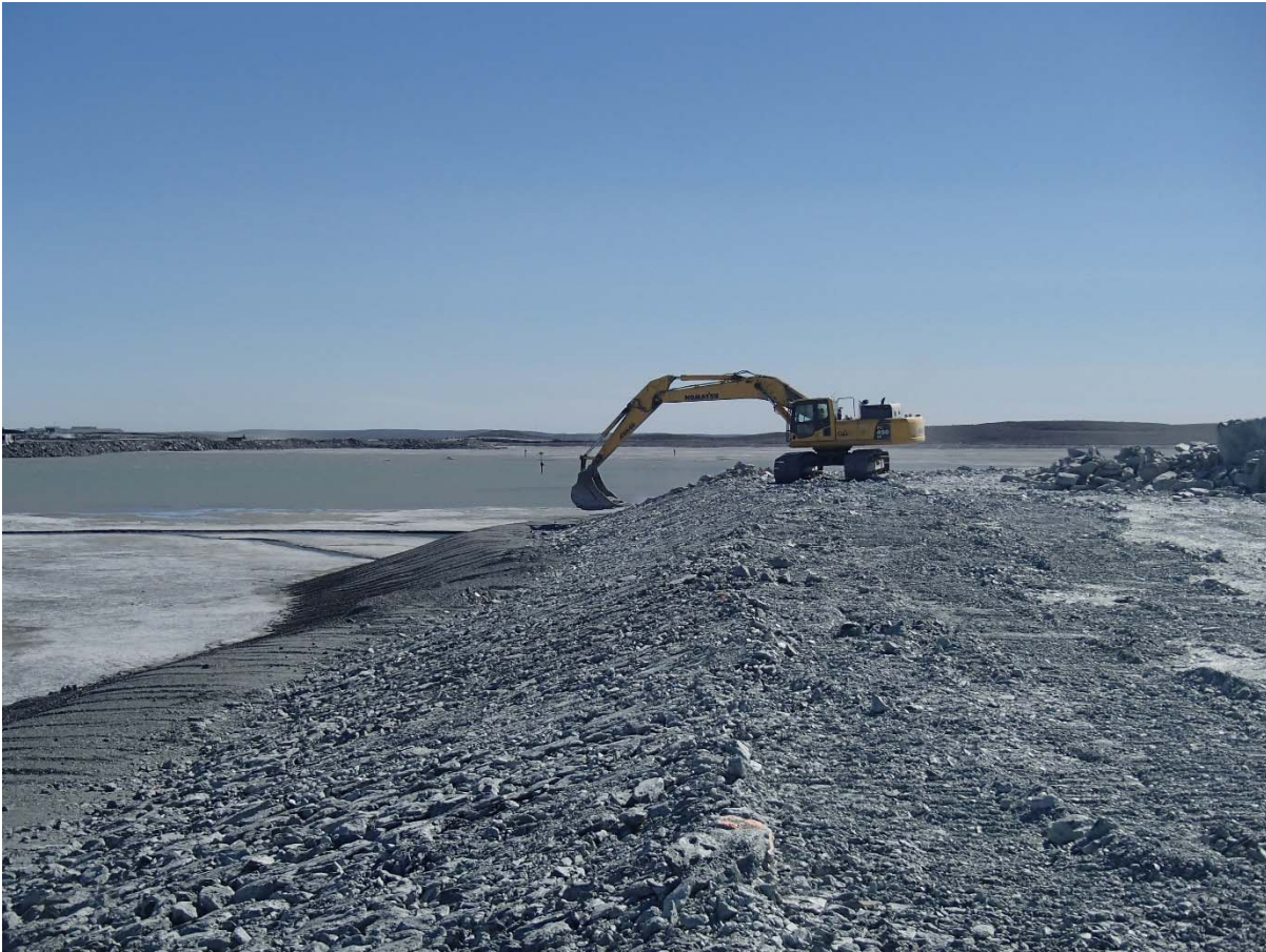
Photograph NCIS-092: From Sta 1+160/-77 m (approx.), looking S. Profiling of the upstream slope (3H:1V) from El. 150 to 152 m with an excavator from Sta. 1+185 m to 1+135 m.
