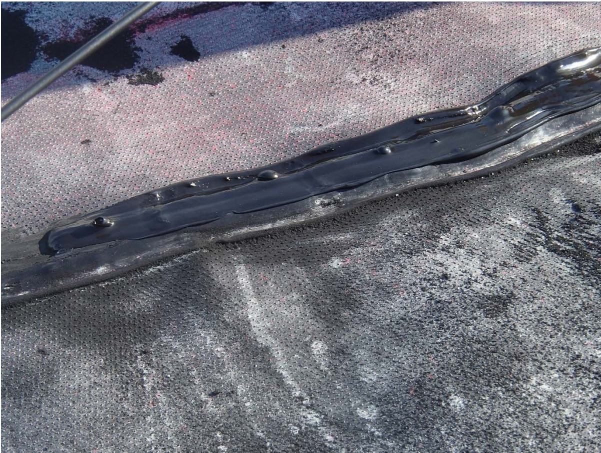
Photograph CD-1864: From Sta. 40+700/-38 m. View of bubbles formed in the extrusion weld because of humidity.
