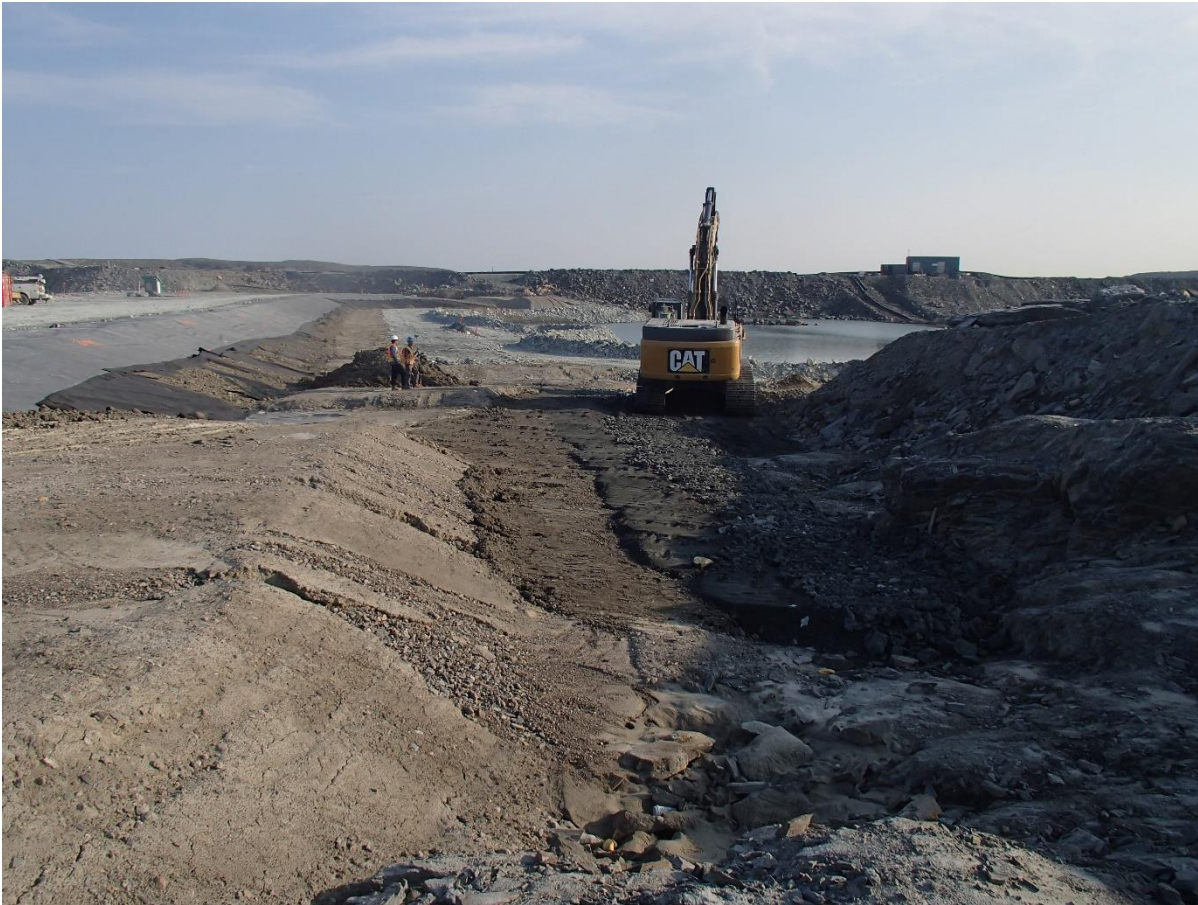
Photograph SD3-326: From Sta. 20+820/-34 m, looking N. Placement of the 0.5 m thick lift of low class till, fine filter, coarse filter and fine rockfill on the upstream slope of the upstream toe liner tie-in with an excavator from Sta. 20+780 to 20+810 m.
