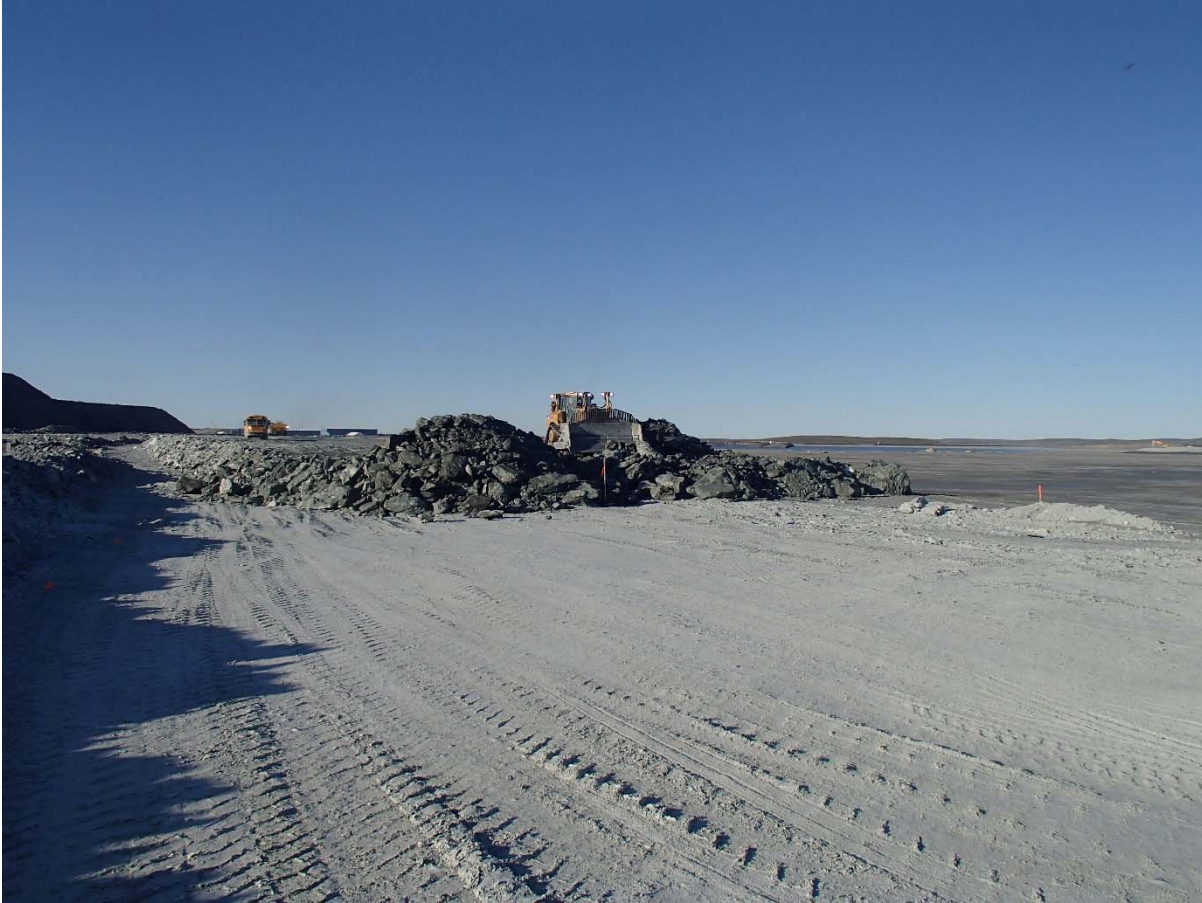
Photograph NCIS-093: From Sta 2+260/+12 m (approx.), looking S. Placement of a 2 m thick (approx.) lift of UM rockfill from El. 152 m to El. 154 m (approx.) with a dozer from Sta. 2+290 m to 2+280 m (+9 m to -22 m).
