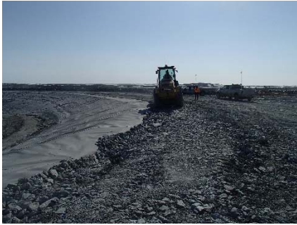
CD-1895 (2018-06-11), looking E from Sta. 40+670/-15 m. Compaction of the geosynthetics tie-in material at El. 145 m with a 10-tonne smooth-drum compactor with vibration (4 passes) from Sta. 40+670 m to 0+950 m.
