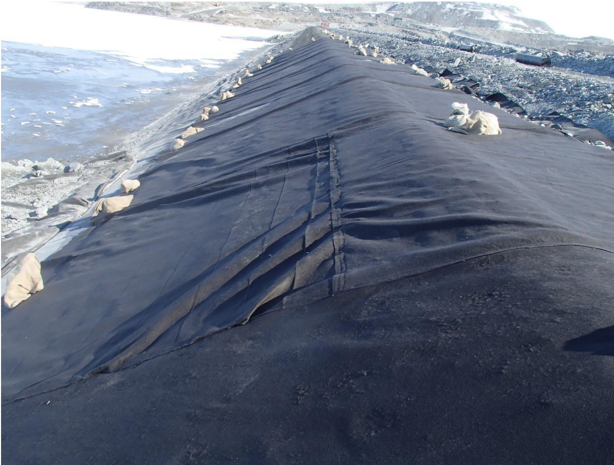
Photograph CD-1881: From Sta. 0+530/-27 m, looking N. View of a geotextile panel with a horizontal weld in the slope at Sta. 0+520 m before its removal.
