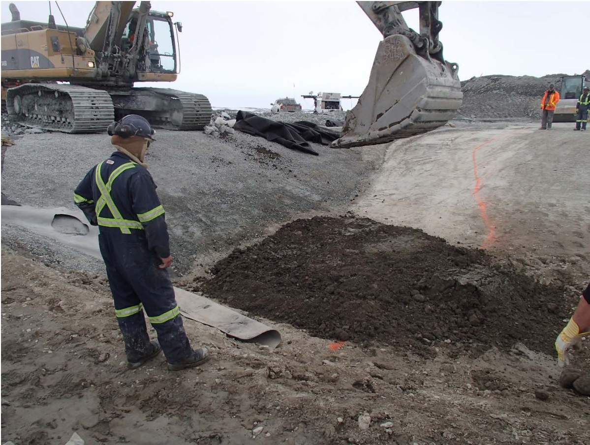
Photograph SD3-312: From Sta. 20+610/-48 m, looking W. Placement of a 0.15 m thick lift of compacted sieved till from Sta. 20+596.4 m to 20+601.6 m (offset -42.6 to -46.3 m) to fill the depression in the compacted sieved till layer.
