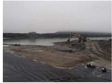
SD3-317 (2018-07-07), looking E from Sta. 20+800/-22 m. Reworking of the access to SD3.
