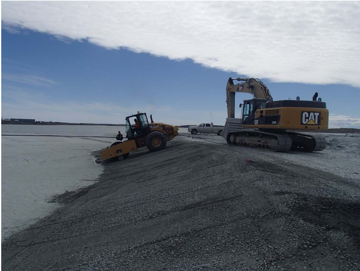
Photograph NCIS-070: From Sta. 1+160/-89 m (approx.), looking S. Compaction of the 0.5 m lift of fine filter between El. 150 and 152 m with a 10-tonne smooth-drum compactor with vibration (4 passes) in the upstream slope from Sta. 1+335 m to 1+100 m.
