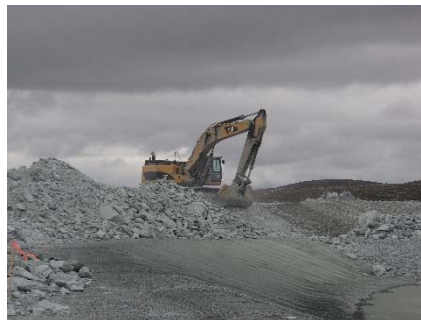
NCIS-134 (2018-07-30), looking NE from Sta. 1+630/-32 m (approx.). Completion of the profiling of the upstream slope (3H:1V) from El. 152 to 154 m with an excavator from Sta. 1+700 m to 1+660 m.
