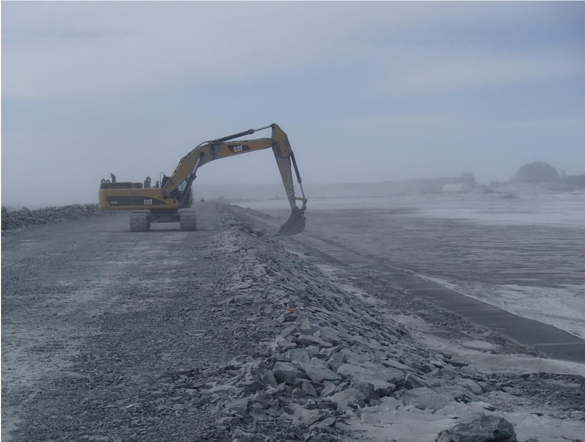
Photograph CD-1816: From Sta. 0+175/-27, looking S. Profiling of the upstream slope (2H:1V) from El. 143 to 145 m with an excavator between Sta. 0+175 and 0+560 m.
