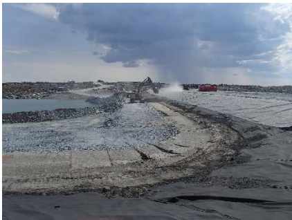
SD3-329 (2018-07-11), looking N from Sta. 20+820/-34 m. Placement of a 0.5 m thick lift of low quality till (0-150 mm) from El. 142.5 m to 143 m from Sta. 20+610 m to 20+760 m.
