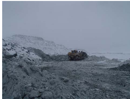
NCIS-005 (2018-05-19). Removal of the excavated material, pushed with a dozer towards the center of the North Cell to clear the upstream toe.
