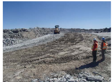
SD3-337 (2018-07-14), looking S from Sta. 20+760/-37 m. Compaction of the fourth 0.5 m thick lifts of fine filter, coarse filter and fine rockfill on the upstream slope of the upstream toe liner tie-in with a 10 tonne smooth-drum compactor with vibrations (4 passes) from Sta. 20+770 to 20+800 m.
