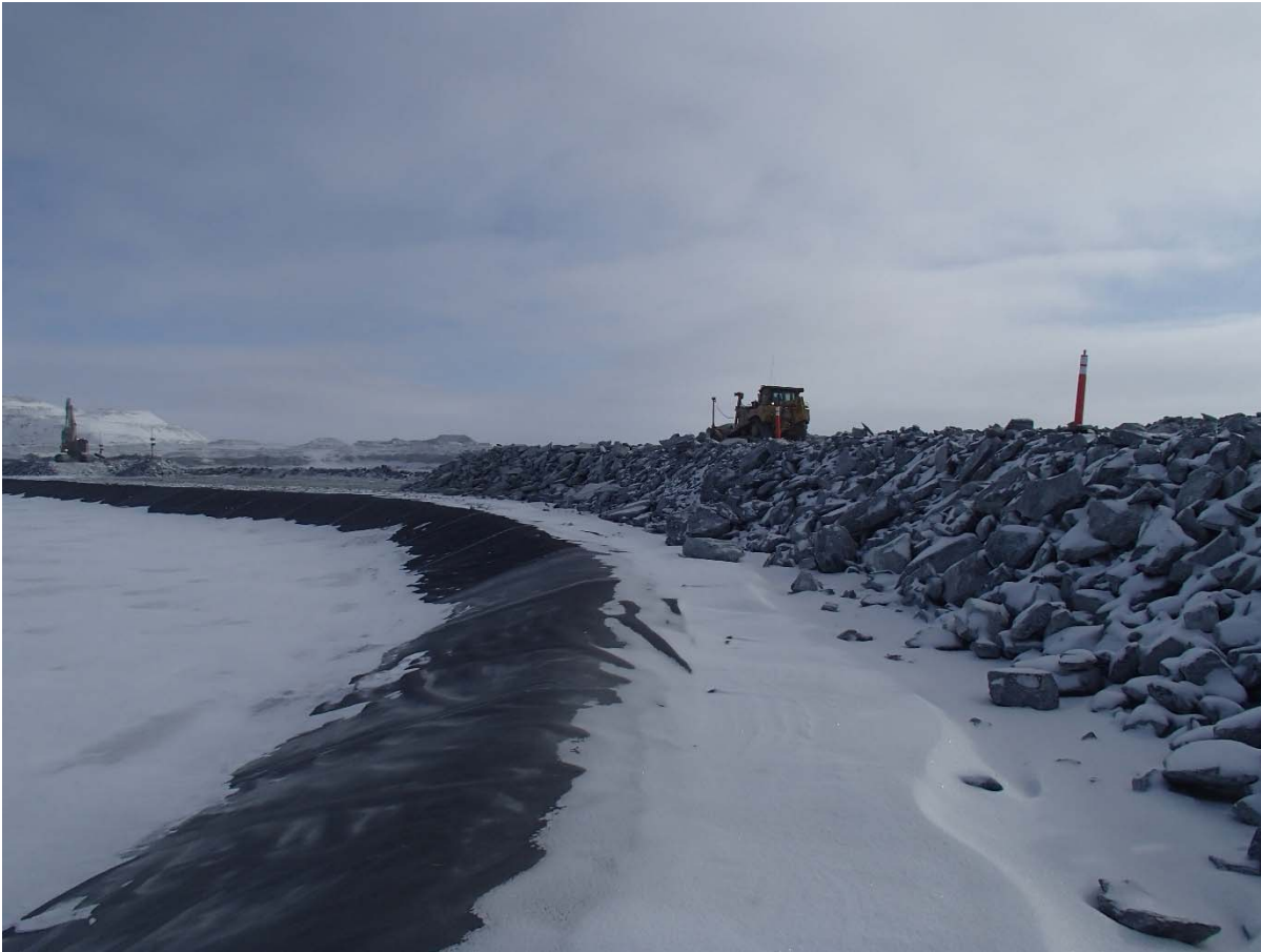
Photograph CD-1818: From Sta. 40+770/-25, looking NE. Placement of a 2 m thick (approx.) lift of intermediate volcanic (IV) rockfill from El. 143 m to El. 145 m from approx. Sta. 0+980 m to 0+880 m (o.s. -28 to -11 m).
