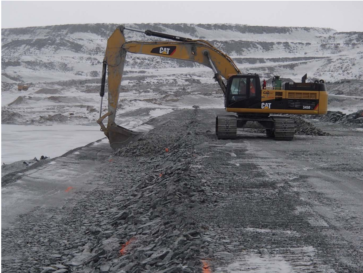
Photograph CD-1841: From Sta. 0+475/-14 m, looking N. Placement of a third 0.5 m thick lift of coarse filter from El. 144 m to 144.5 m with an excavator from Sta. 0+335 m to 40+730 m.
