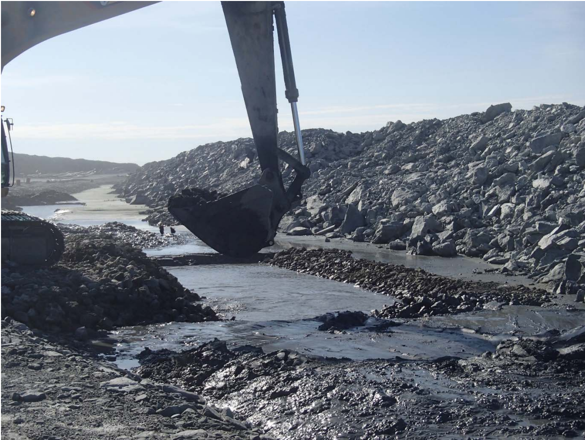
Photograph NCIS-124: From Sta. 3+340/+33 m (approx.), looking S. Placement of a 0.3 m thick (approx.) layer of till sieving reject material on the bottom and on the slopes of the south sump.
