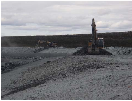
NCIS-109 (2018-07-22), looking N from Sta. 2+450/-21 m (approx.). Placement of a 0.5 m thick lift of coarse filter in the upstream slope from El. 152 m to 154 m with an excavator from Sta. 2+293 m to 2+411 m.
