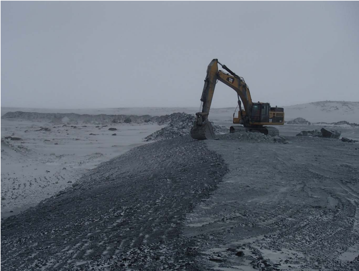
Photograph NCIS-019: From Sta. 2+100 m (approx.), looking SW. Profiling of the upstream slope (3H:1V) from El. 150 to 152 m with an excavator from Sta. 1+860 m to 1+678 m. The portion between Sta. 1+900 m and 1+800 m, where the structure is built on the natural ground, was not profiled.
