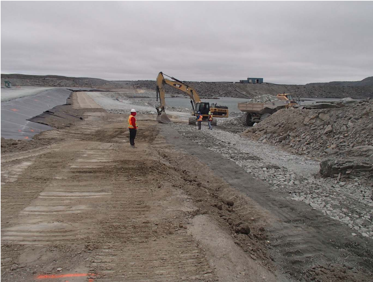
Photograph SD3-333: From Sta. 20+817/-29 m, looking N. Placement of a second 0.5 m thick lift of fine rockfill on the upstream slope of the upstream toe liner tie-in with an excavator from Sta. 20+775 m to 20+800 m.
