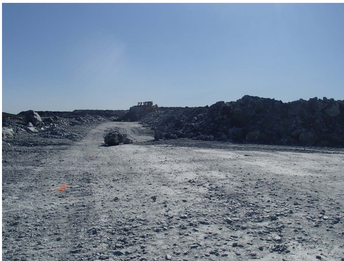
Photograph NCIS-100: From Sta. 1+960/+10 m (approx.), looking E. Placement of a 2 m thick (approx.) lift of UM rockfill from El. 152 m to El. 154 m (approx.) with a dozer from Sta. 1+984 m to 1+947 m (+14 m to -26 m). The material is of good quality and is well graded.
