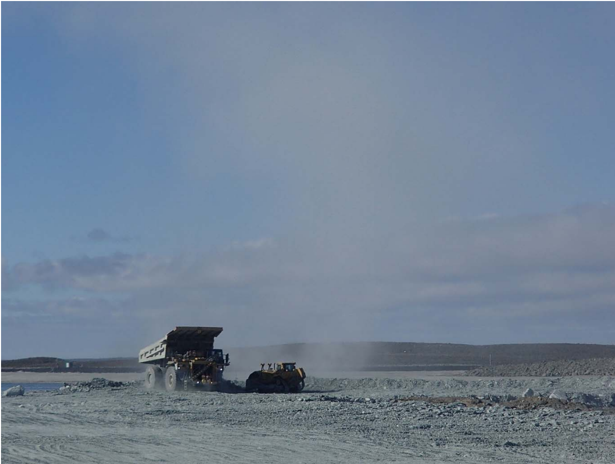
Photograph NCIS-059: From Sta. 1+330/-34 m (approx.), looking S. Placement of a 1.5 to 2 m thick (approx.) lift of UM rockfill from El. 148 m to El. 150 m (approx.) with a dozer from Sta. 1+120 m to 1+100 m (-96 m to -60 m). The material is of good quality and is well graded.
