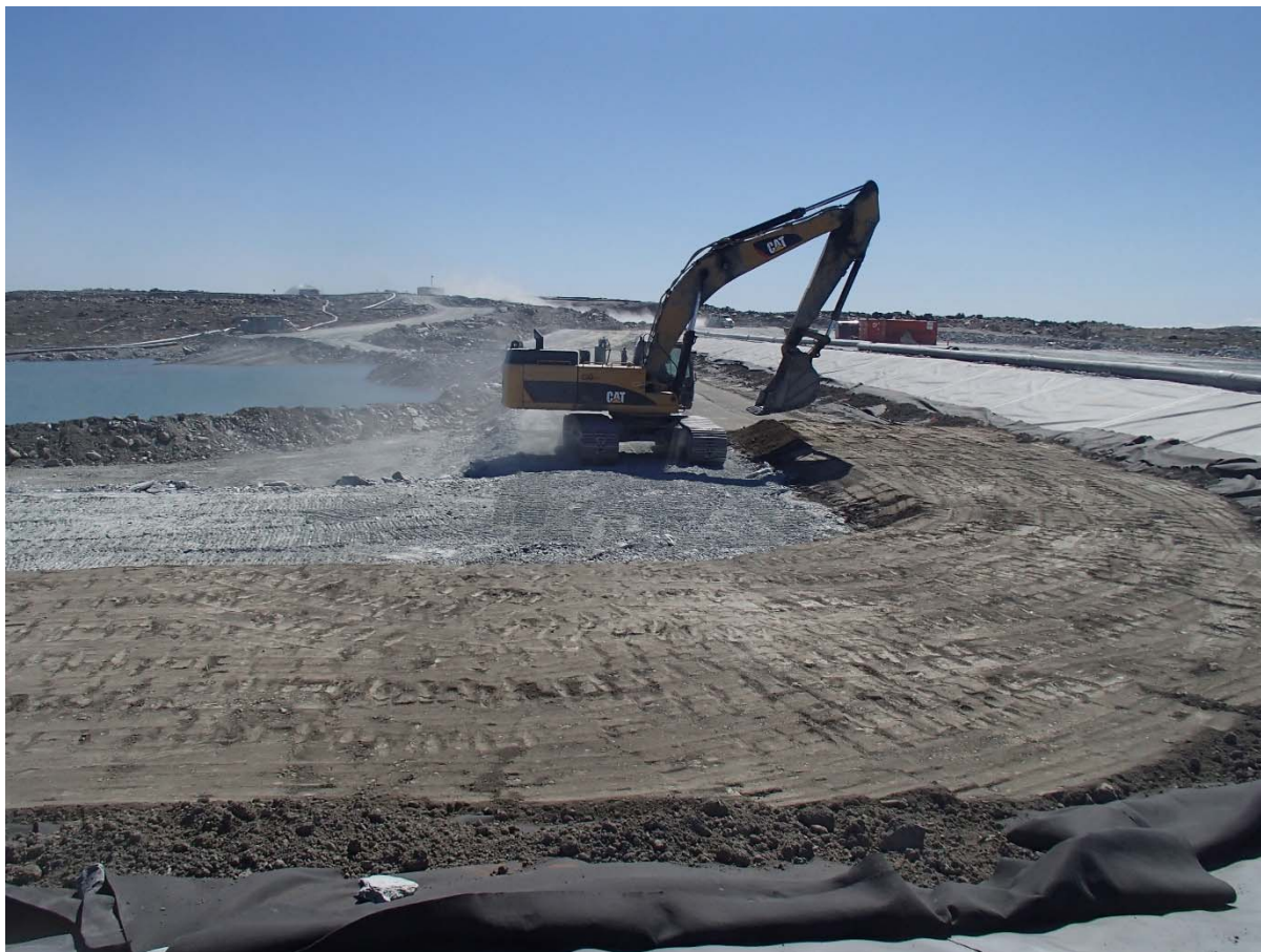
Photograph SD3-344: From Sta. 20+610/-43 m, looking S. Placement of a third 0.5 m thick lift of low quality till (0-150 mm) from El. 142.5 m to 143 m from Sta. 20+570 m to 20+590 m.
