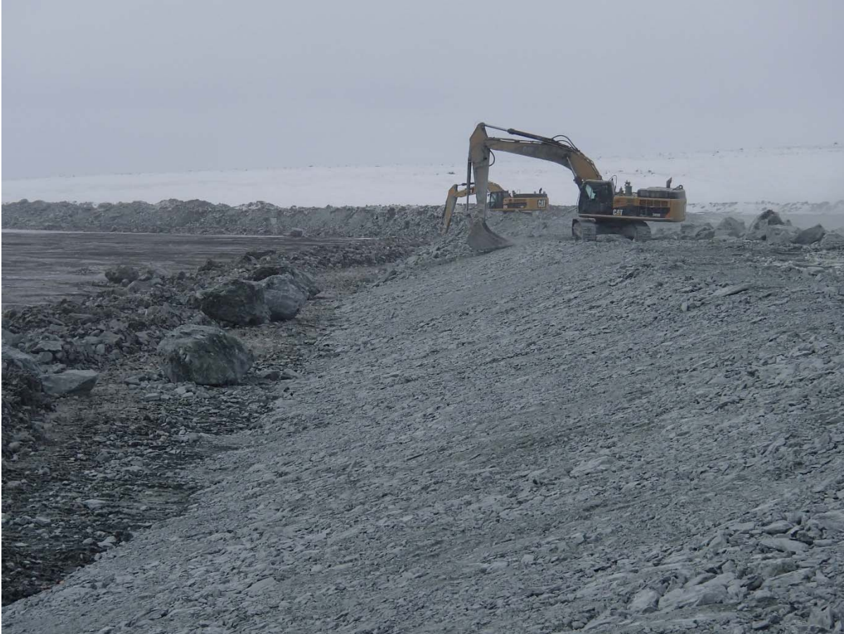
Photograph NCIS-007: Profiling of the upstream slope (3H:1V) from El. 150 to 152 m with an excavator.
