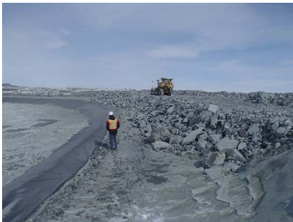
CD-1817 (2018-05-02), looking NE from Sta. 40+700/-10 m. View of the rockfill lift thickness at the junction of Saddle Dam 5 and Central Dike, approx. 2.5 m thick..
