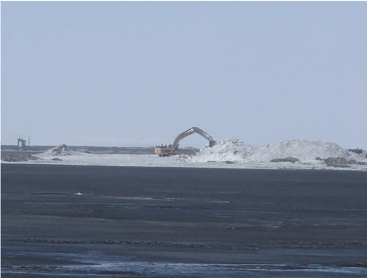
Photograph NCIS-024: From Sta. 2+570 m (approx.), looking SW. Removal of the snow bank in the footprint with an excavator from Sta. 1+160 m to 1+120 m (approx.).
