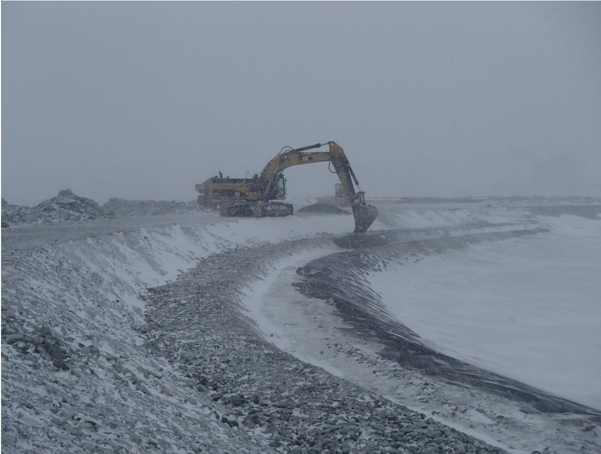
Photograph CD-1827: From Sta 0+940/-16 m, looking SW. Placement of a 0.5 m thick lift of fine filter from El. 143 m to 143.5 m with an excavator from Sta. 40+730 m to 0+ 835 m.
