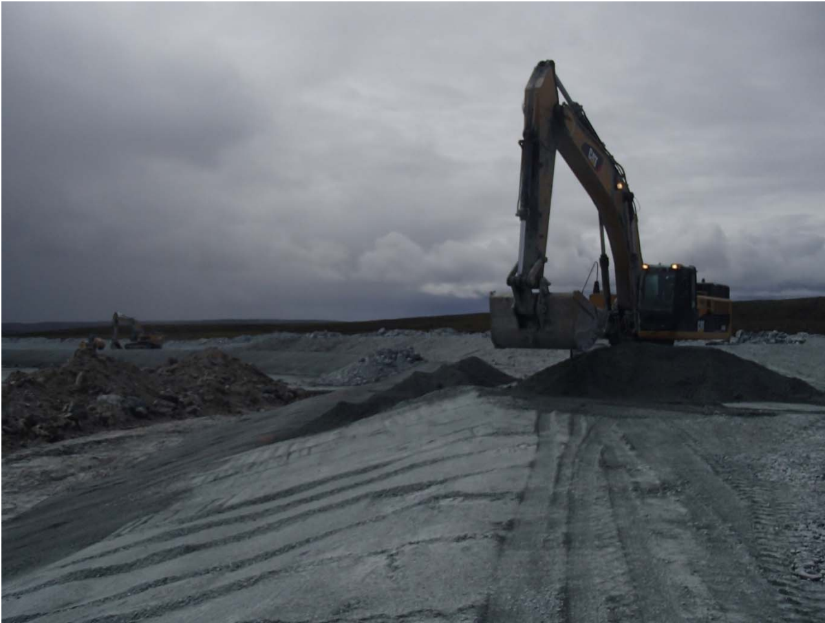
Photograph NCIS-135: From Sta. 1+860/-12 m (approx.), looking SW. Placement of a 0.5 m thick lift of fine filter in the upstream slope from El. 152 m to 154 m with an excavator from Sta. 1+830 m to 1+700 m.
