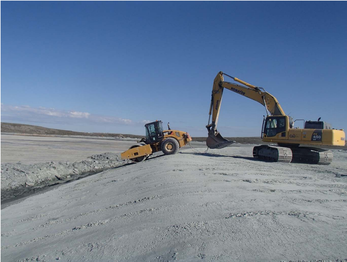
Photograph NCIS-112: From Sta. 2+610/-29 m (approx.), looking N. Compaction of the 0.5 m lift (approx.) of coarse filter between El. 152 m and 154 m with a 10-tonne smooth-drum compactor with vibration (4 passes) in the upstream slope from Sta. 2+080 m to 2+000 m.
