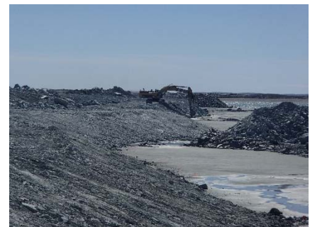
NCIS-072 (2018-07-02), looking W from Sta. 2+790/-38 m. Profiling of the upstream slope (3H:1V) from El. 150 to 152 m with an excavator from Sta. 2+975 m to 3+070 m.
