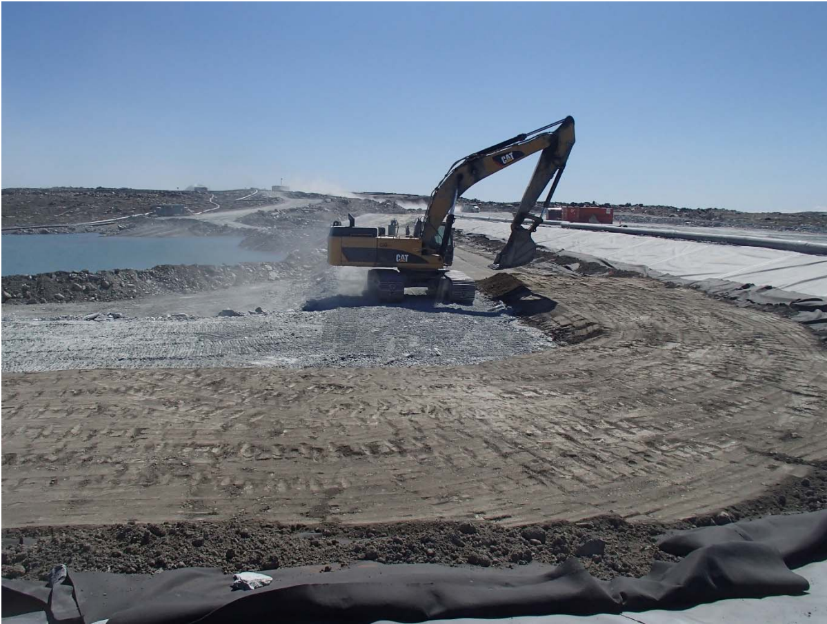
Photograph SD3-344: From Sta. 20+610/-43 m, looking S. Placement of a third 0.5 m thick lift of low quality till (0-150 mm) from El. 142.5 m to 143 m from Sta. 20+570 m to 20+590 m.
