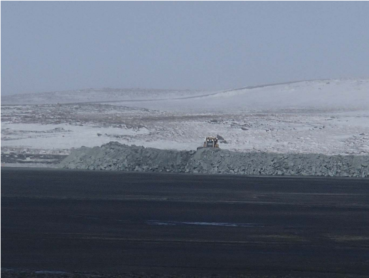
Photograph NCIS-023: From Sta. 2+570 m (approx.), looking W. Placement of a 2 m thick (approx.) lift of UM rockfill from El. 150 m to El. 152 m (approx.) with a dozer from Sta. 1+500 m to 1+450 m (offset unavailable). The material is of good quality and is well graded.
