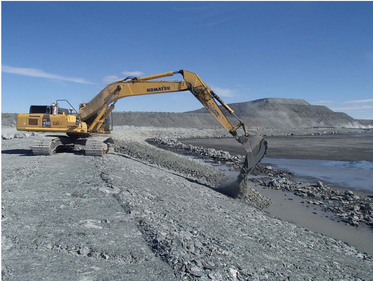
Photograph NCIS-029: From Sta. 2+120/-27 m (approx.), looking SE. Placement of a 0.5 m thick lift of coarse filter in the upstream slope from El. 150 m to 152 m with an excavator from Sta. 2+280 m to 2+105 m.
