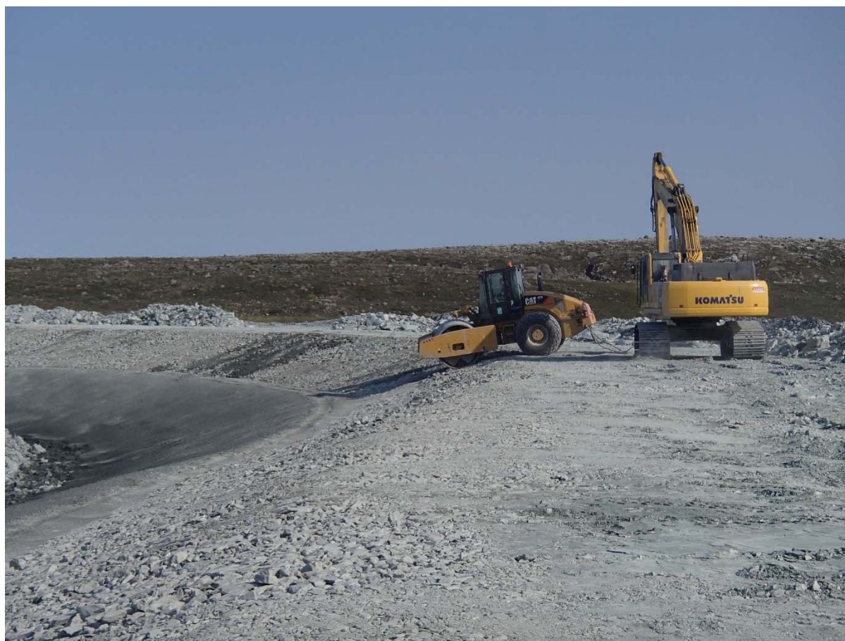
Photograph NCIS-110: From Sta. 2+320/-22 m (approx.), looking N. Compaction of the 0.5 m lift (approx.) of coarse filter between El. 152 m and 154 m with a 10-tonne smooth-drum compactor with vibration (4 passes) in the upstream slope from Sta. 2+293 m to 2+080 m.
