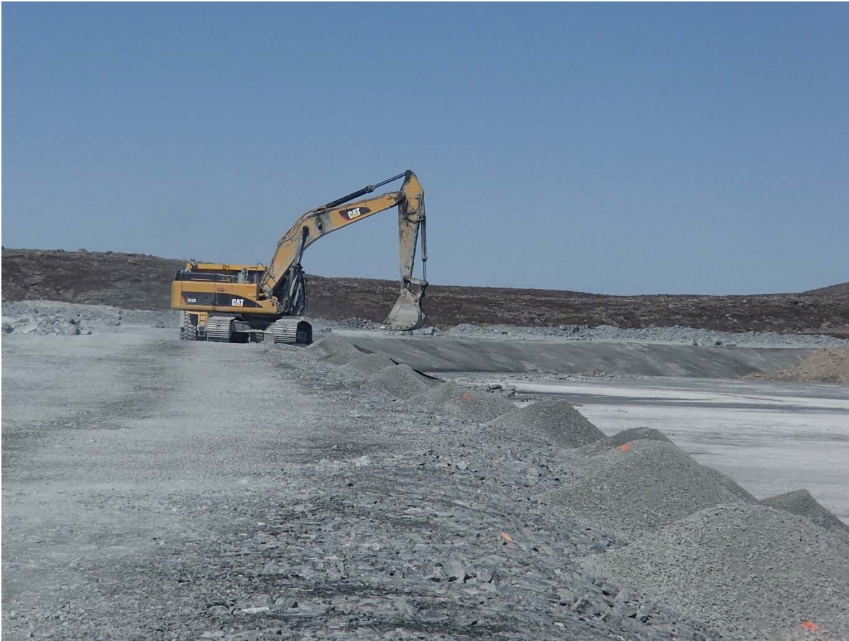
Photograph NCIS-066: From Sta. 1+400/-34 m (approx.), looking N. Placement of a 0.5 m thick lift of fine filter over the coarse filter in the upstream slope from El. 150 m to 152 m with an excavator from Sta. 1+595 m to 1+550 m.
