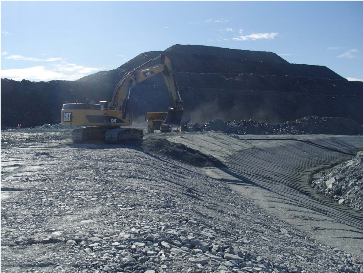
Photograph NCIS-104: From Sta. 2+650/-23 m (approx.), looking SE. Placement of a 0.5 m thick lift of fine filter in the upstream slope from El. 152 m to 154 m with an excavator from Sta. 2+710 m to 2+445 m.
