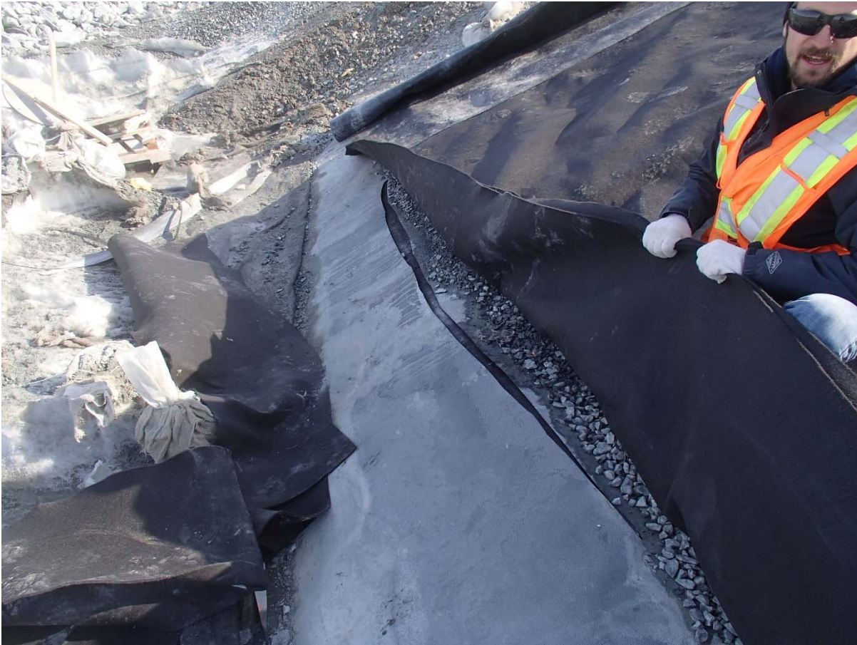
Photograph CD-1889: From Sta. 0+150/-28 m, looking N. View of the underlying liner that has been cut at around Sta. 0+160 m to drain the water.
