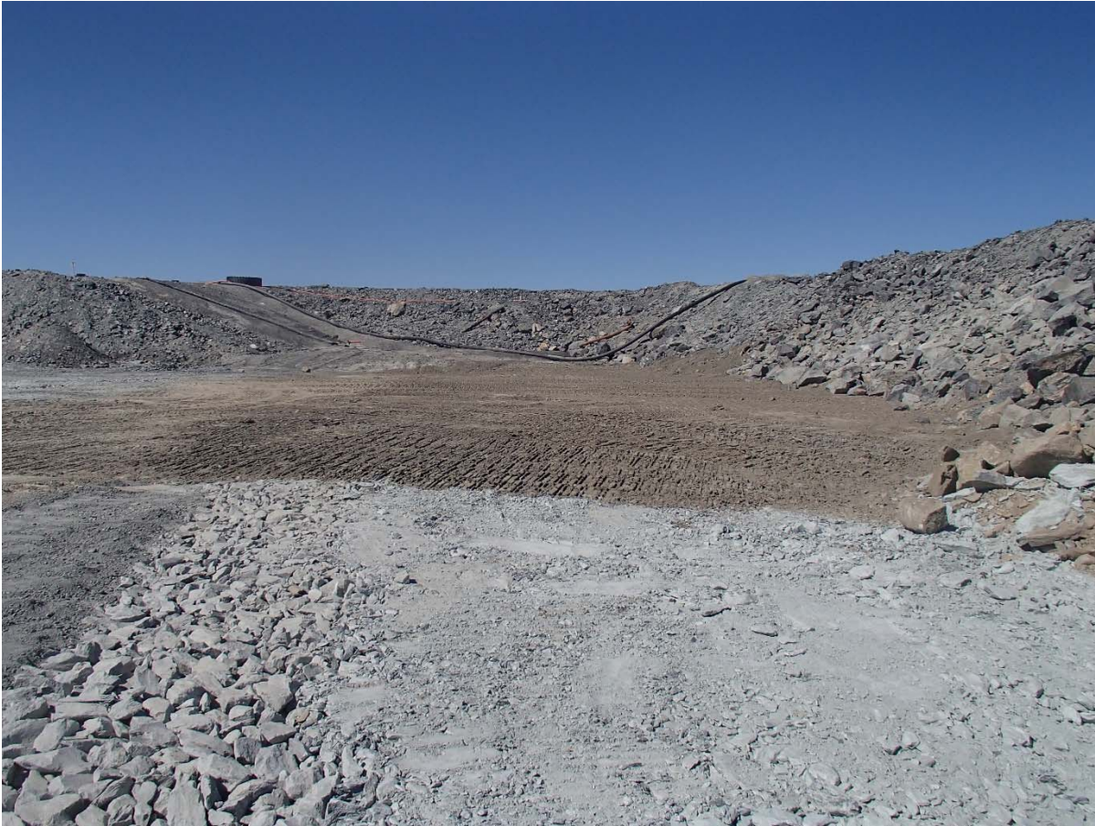
Photograph SD3-343: From Sta. 20+590/-40 m, looking NW. View of the depression between SD2 and SD3 backfilled with low quality till up to El. 145 m.
