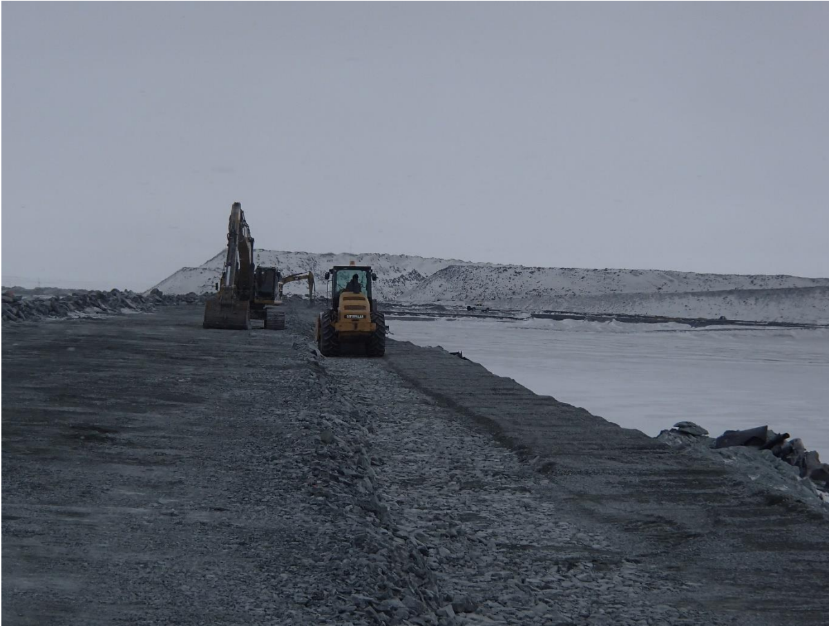
Photograph CD-1843: From Sta 0+460/-23 m, looking S. Compaction of the third 0.5 m lift (approx.) of fine and coarse filters material at El. 144.5 m with a 10-tonne smooth-drum compactor with vibration (4 passes) from Sta 0+335m to 0+900 m.
