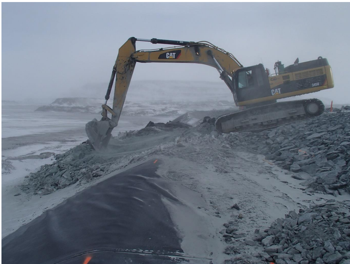
Photograph CD-1830: From Sta 0+420/-26 m, looking N. Removal of the deposition point finger materials with an excavator at Sta. 0+390 m.
