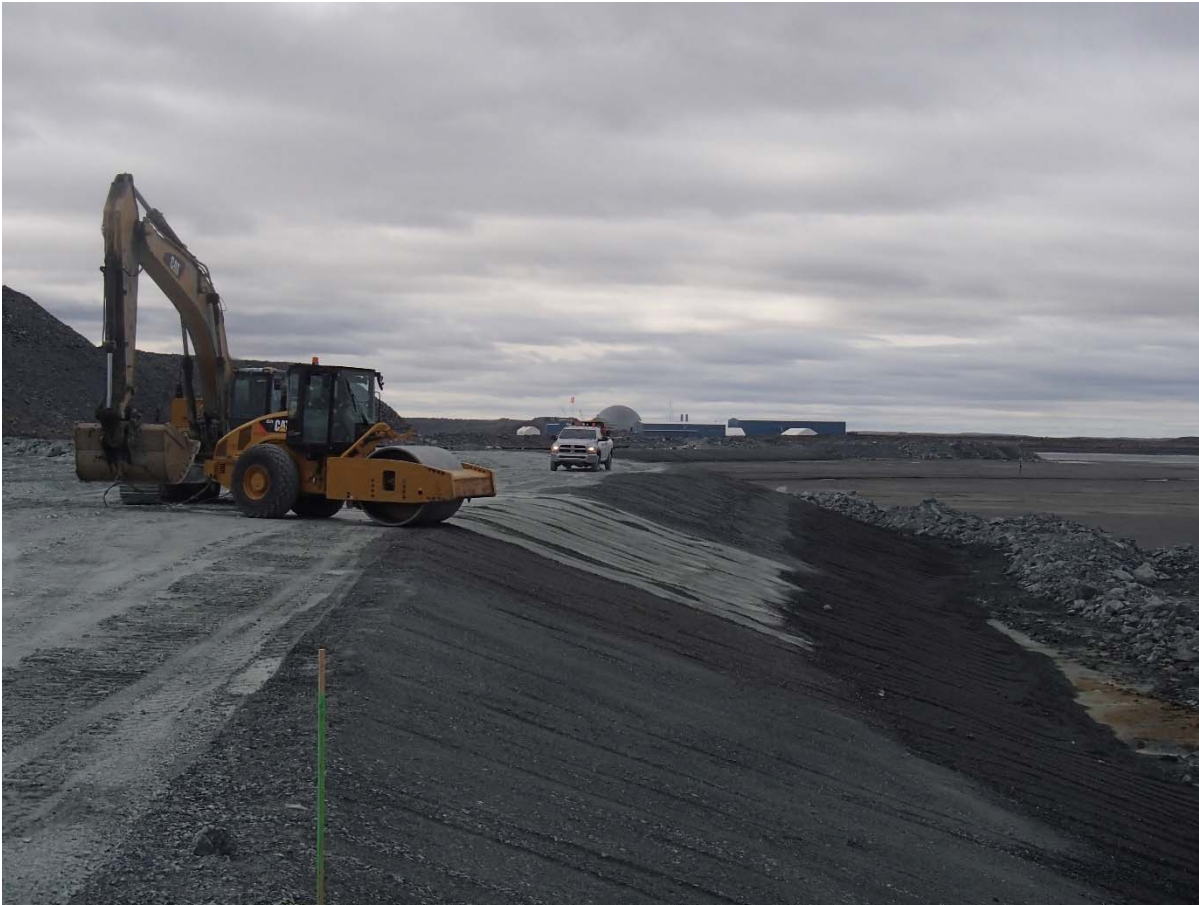
Photograph NCIS-129: From Sta. 2+450/-21 m (approx.), looking S. Compaction of the 0.5 m lift (approx.) of fine filter between El. 152 m and 154 m with a 10-tonne smooth-drum compactor with vibration (4 passes) in the upstream slope from Sta. 2+220 m to 1+940 m.
