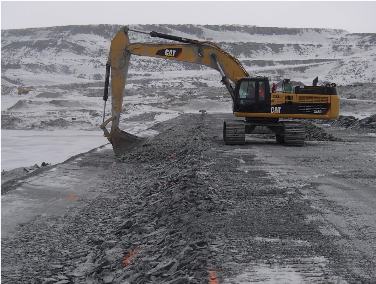
Photograph CD-1841: From Sta 0+475/-14 m, looking N. Placement of a third 0.5 m thick lift of coarse filter from El. 144 m to 144.5 m with an excavator from Sta. 0+335 m to 40+730 m.
