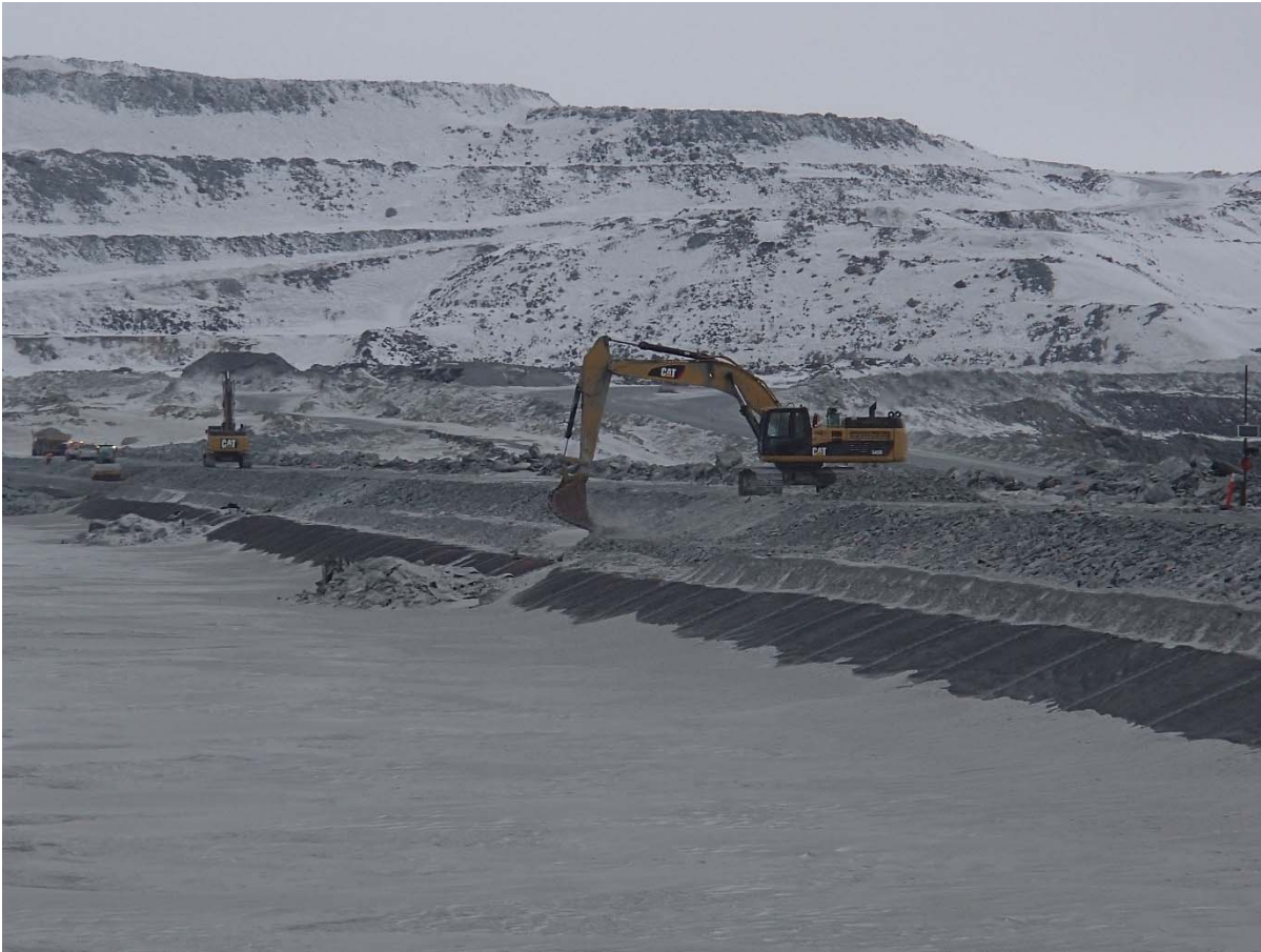
Photograph CD-1834: From Sta. 40+760/-23 m, looking NE. Placement of a first 0.5 m thick lift of coarse filter from El. 143 m to 143.5 m on length of approx. 5 m with an excavator at the location of the deposition finger at Sta. 0+520 m and 0+660 m.
