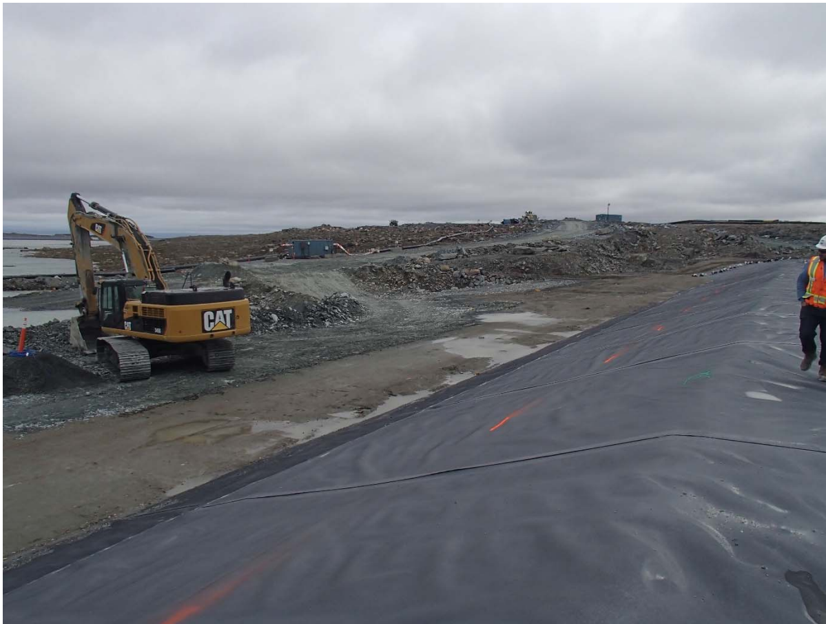
Photograph SD3-318: From Sta. 20+710/-24 m, looking SE. Placement of IV rockfill in the water up to El. 142 m with an excavator from Sta. 20+785 m to 20+730 m, at the bottom of the upstream slope of SD3 to widen the rockfill layer and allow access to the erosion protection.
