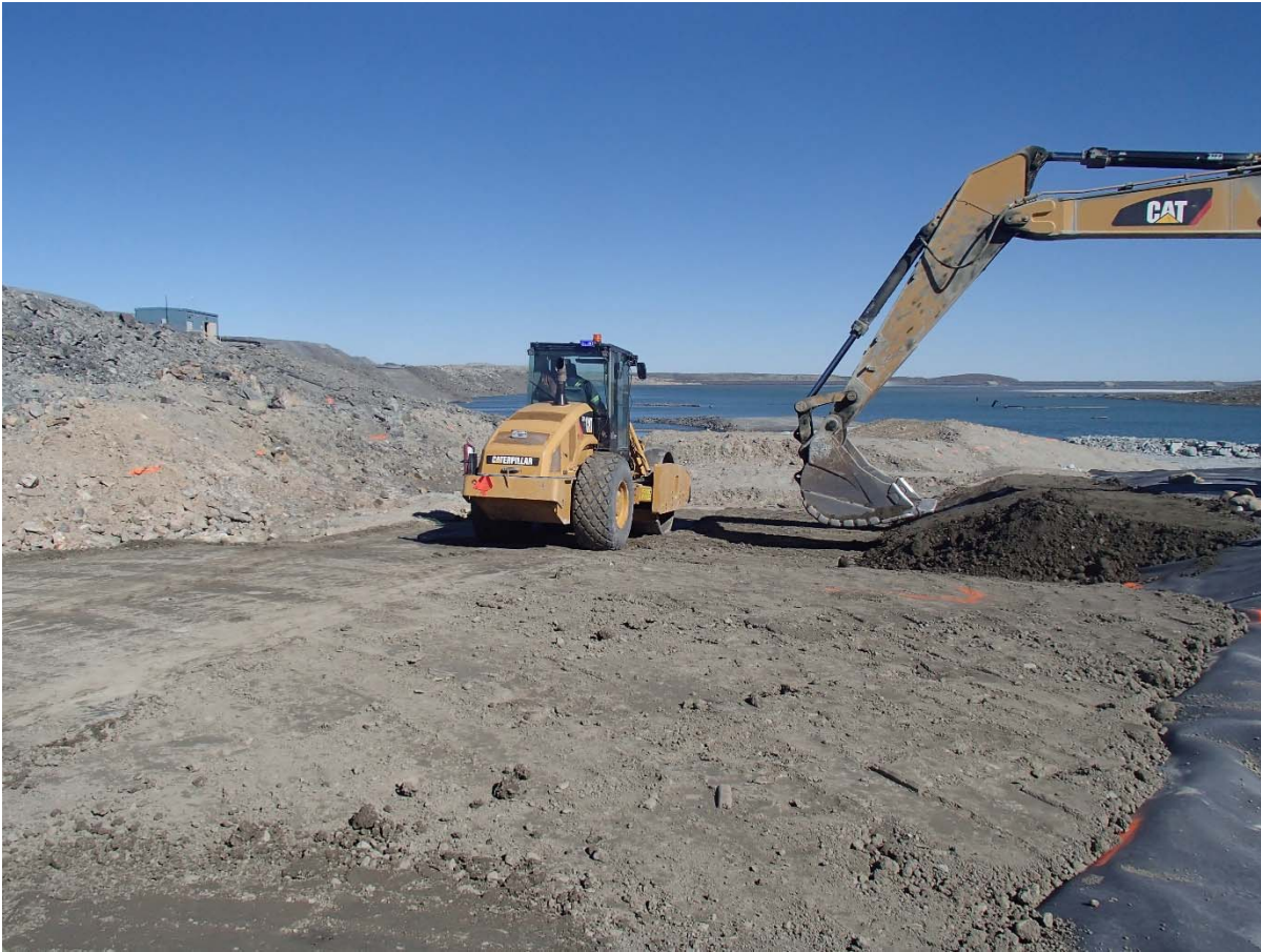
Photograph SD3-339: From Sta. 20+600/-29 m, looking E. Compaction of a first 0.5 m thick lift of compacted sieved till on the upstream toe liner tie-in with an excavator from Sta. 20+588 m to 20+599 m.
