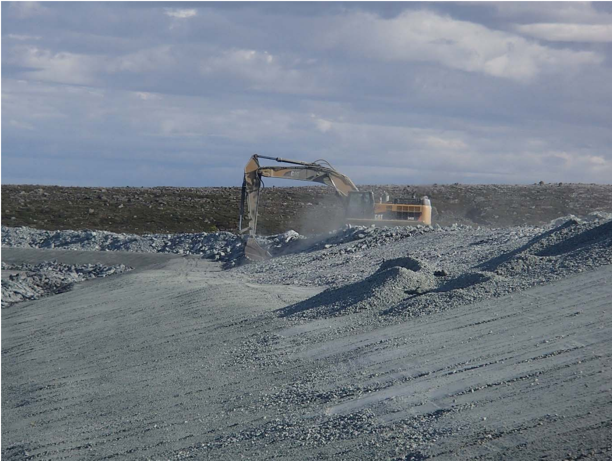
Photograph NCIS-108: From Sta. 2+490/-32 m (approx.), looking N. Profiling of the upstream slope (3H:1V) from El. 152 to 154 m with an excavator from Sta. 2+159 m to 2+409 m.
