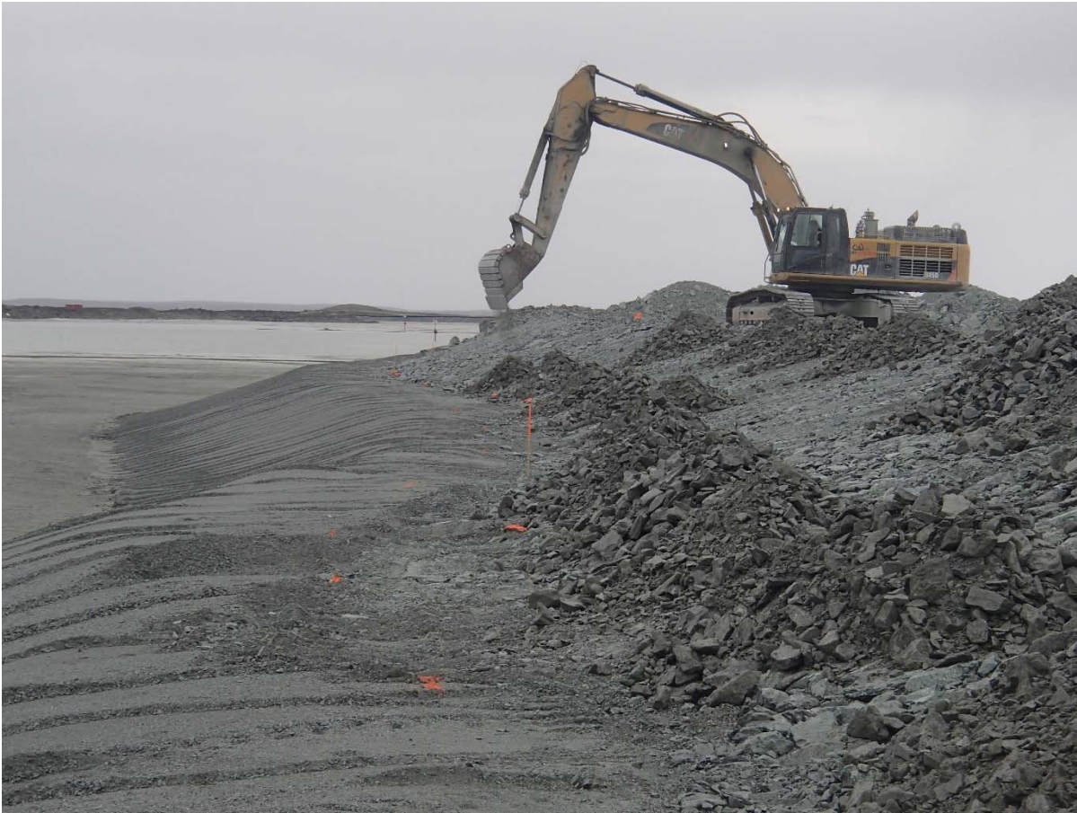
Photograph NCIS-079: From Sta. 1+280/-39 m (approx.), looking SW. Placement of a 0.5 m thick lift of coarse filter in the upstream slope from El. 150 m to 152 m with an excavator from Sta. 1+300 m to 1+200 m.
