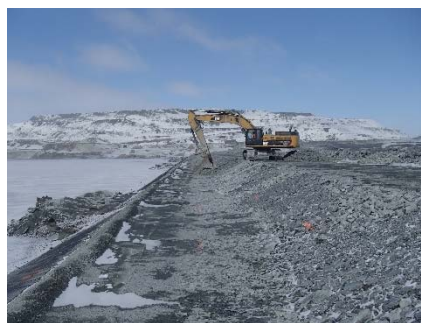
CD-1839 (2018-05-09), looking N from Sta. 0+835/-20 m. Placement of a second 0.5 m thick lift of coarse filter from El. 143.5 m to 144 m with an excavator from Sta. 0+500 m to 0+835 m and from 0+930 to 40+730 m.
