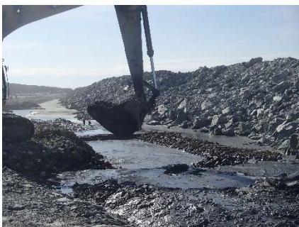
NCIS-124 (2018-07-27), looking S from Sta. 3+340/+33 m (approx.). Placement of a 0.3 m thick (approx.) layer of till sieving reject material on the bottom and on the slopes of the south sump.
