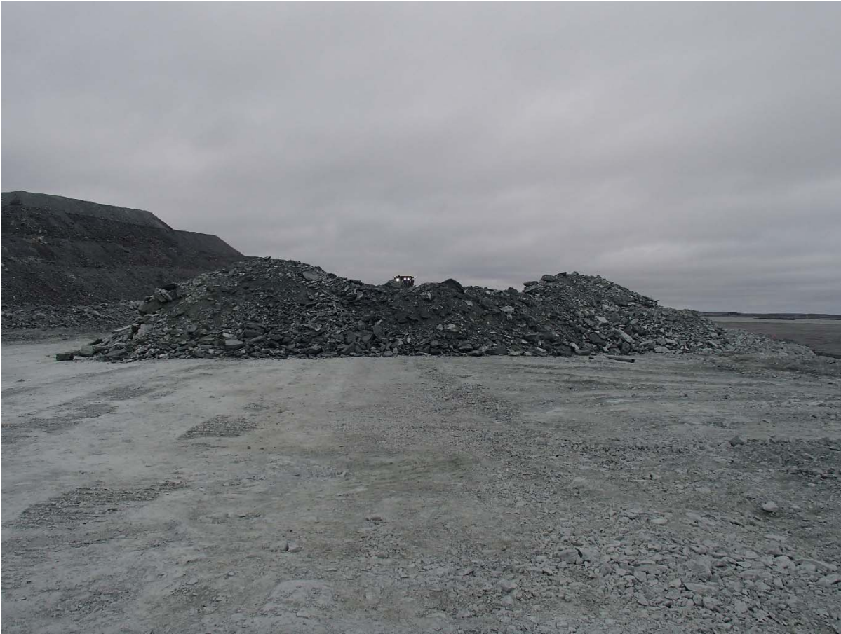
Photograph NCIS-090: From Sta 2+440/-1 m (approx.), looking SE. Placement of a 2 m thick (approx.) lift of UM rockfill from El. 152 m to El. 154 m (approx.) with a dozer from Sta. 2+455 m to 2+370 m (+4 m to -24 m).
