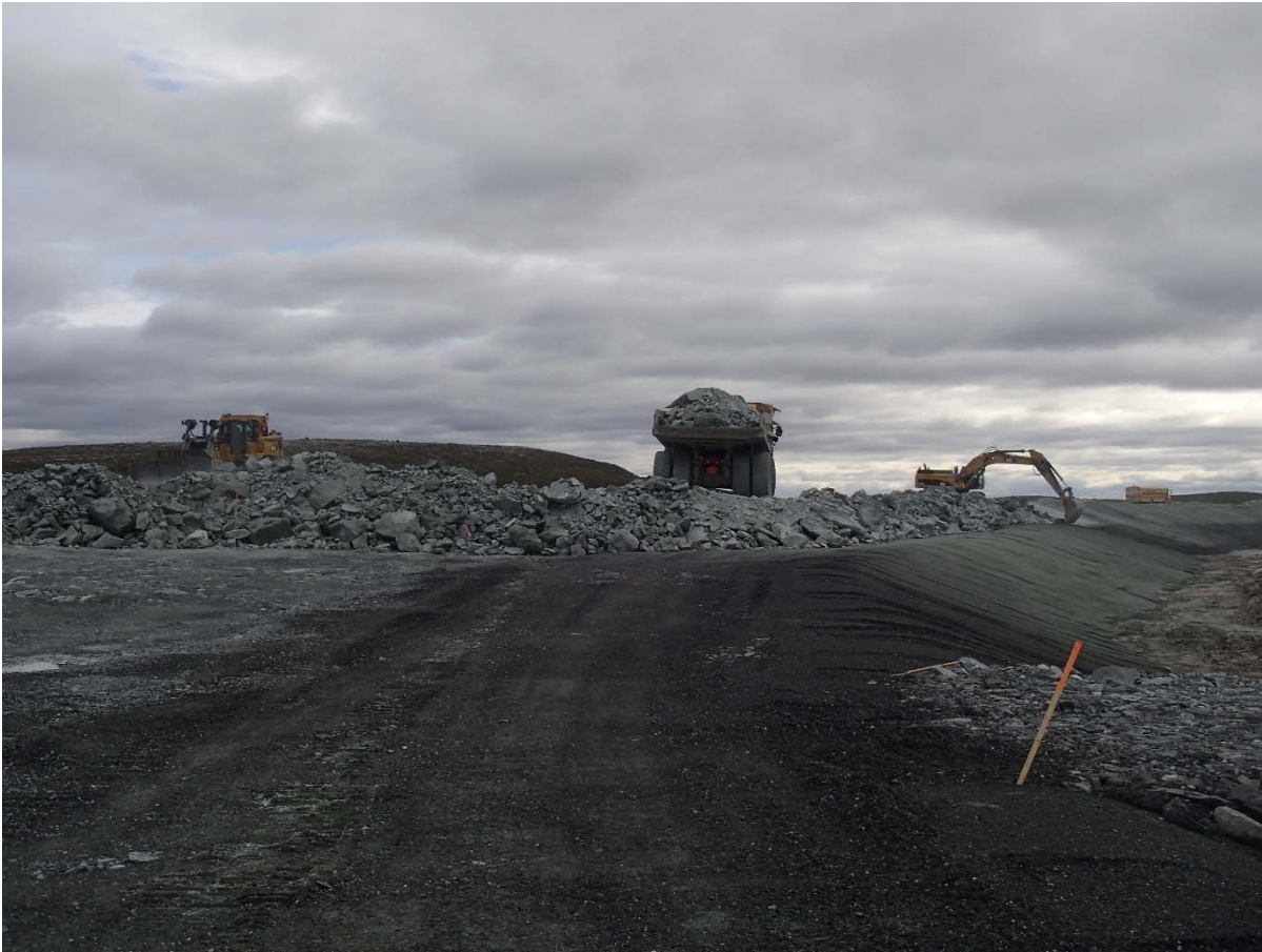
Photograph NCIS-128: From Sta. 1+680/-42 m (approx.), looking NE. Placement of a 2 m thick (approx.) lift of UM rockfill from El. 152 m to El. 154 m (approx.) with a dozer from Sta. 1+830 m to 1+660 m (+8 m to -31 m) and profiling of the upstream slope (3H:1V) from El. 152 to 154 m with an excavator from Sta. 1+880 m to 1+780 m.
