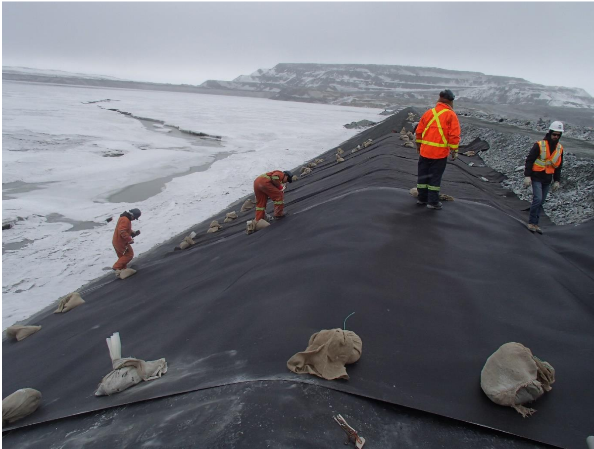
Photograph CD-1874: From Sta. 0+760/-26 m, looking N. Installation of the geotextile on the upstream slope 2H:1V between El. 143 m and 145 m from Sta. 0+760 m to 0+740 m.
