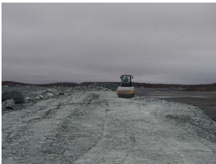
NCIS-043 (2018-06-25), looking N from Sta. 1+250/-38 m. Compaction of the 1.5 to 2 m lift (approx.) of ultramafic (UM) rockfill at El. 150 m with a 10-tonne smooth-drum compactor with vibration (6 passes) between the haul truck traffic lane and the upstream slope from Sta. 1+330 to 1+200 m (o.s. -53 to -24 m).
