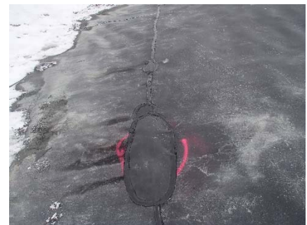
CD-1876 (2018-05-30), looking N from Sta. 0+820/-26 m. View of repair patches on the extrusion weld at the bottom of the panel 838.
