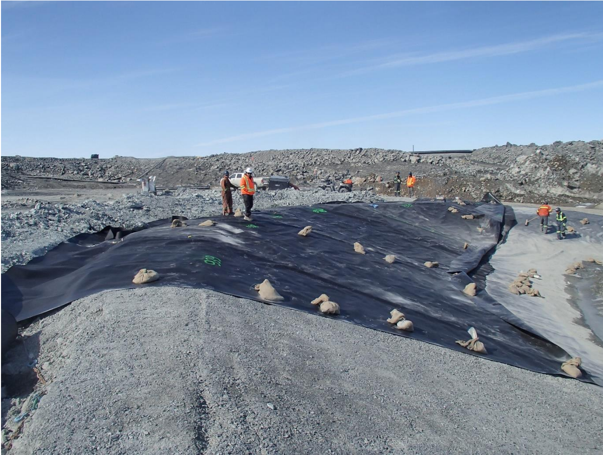
Photograph SD-309: From Sta. 20+640/-26 m, looking N. Installation of the LLDPE liner on the upstream slope 2H:1V between El. 143 m and 145 m from Sta. 20+620 m to 20+630 m (panel numbers 934 to 939).
