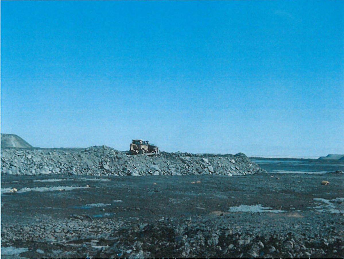
Photograph NCIS-025: From Sta. 1+475 m (approx.), looking SE. Placement of a 2 m thick (approx.) lift of UM rockfill from El. 150 m to El. 152 m (approx.) with a dozer from Sta. 1+450 m to 1+390 m (offset unavailable). The material is of good quality and is well graded.
