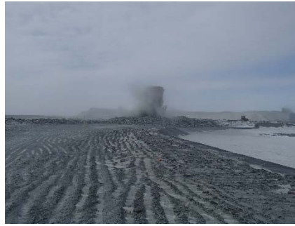
CD-1815 (2018-05-02), looking S from Sta. 0+920/-25 m. Placement of a 2 m thick (approx.) lift of intermediate volcanic (IV) rockfill from El. 143 m to El. 145 m from approx. Sta. 40+740 to 0+980 m (o.s. -28 to -11 m).
