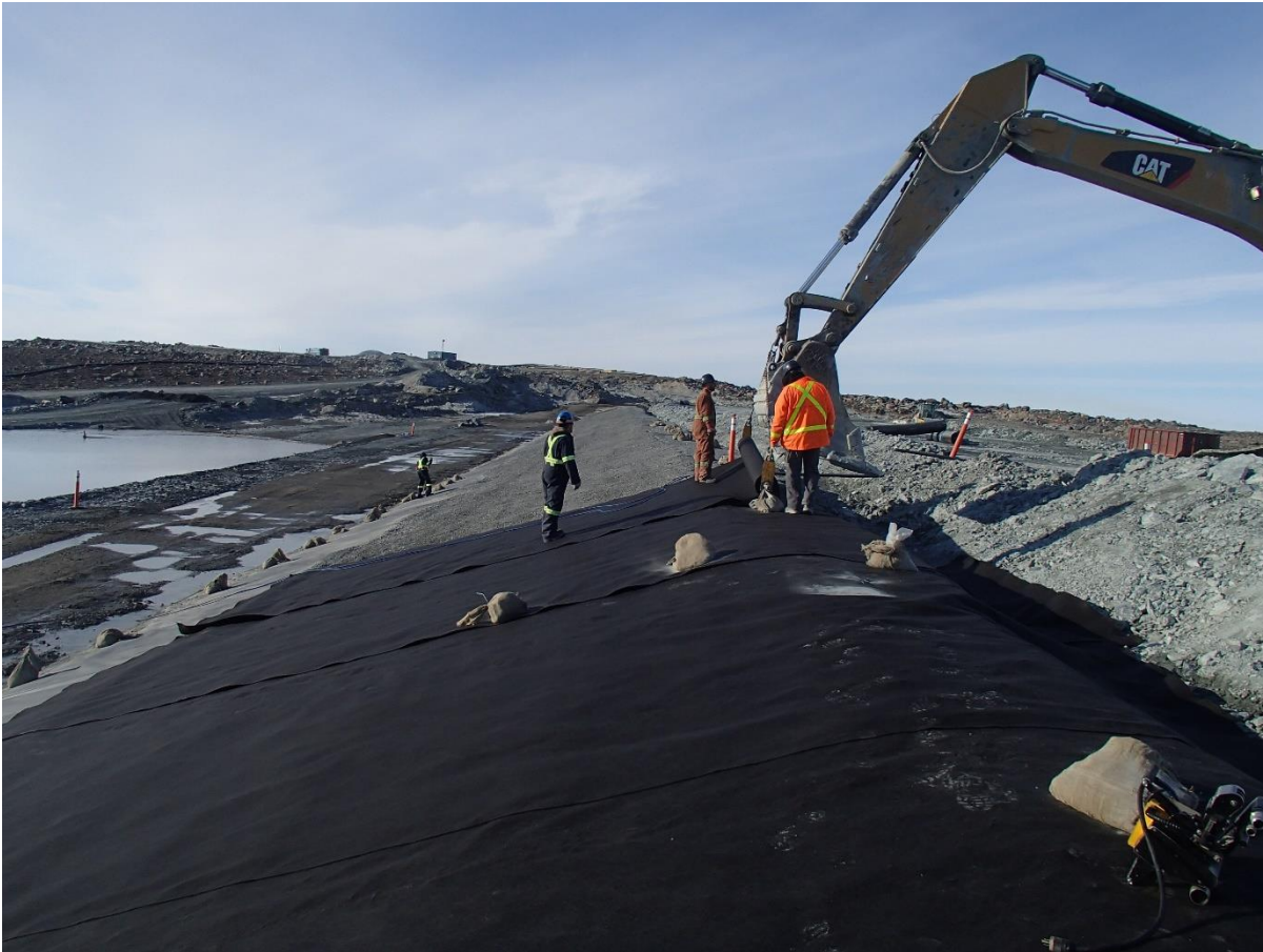
Photograph SD-310: From Sta. 20+635/-24 m, looking S. Installation of the geotextile on the upstream slope 2H:1V between El. 143 m and 145 m from Sta. 20+630 m to 20+800 m.
