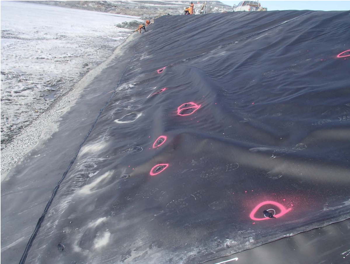
Photograph CD-1879: From Sta. 0+735/-28 m, looking N. View of the repaired holes on panel 850.
