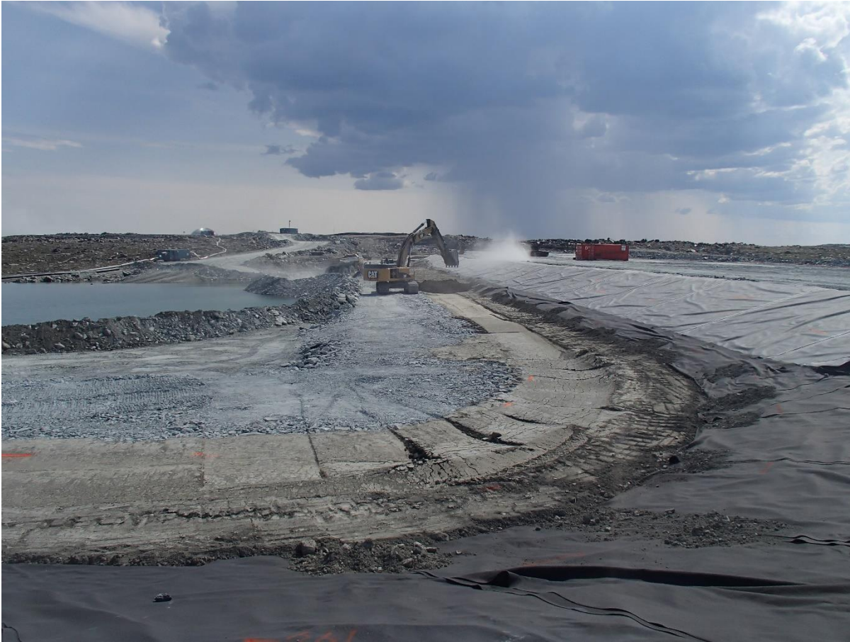
Photograph SD3-329: From Sta. 20+610/-43 m, looking S. Placement of a 0.5 m thick lift of low quality till (0-150 mm) from El. 142.5 m to 143 m from Sta. 20+610 m to 20+760 m.
