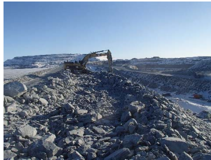
CD-1854 (2018-05-15), looking N from Sta. 0+860/-13 m. Profiling of the downstream slope (1.5H:1V) from El. 143 to 145 m with an excavator between Sta. 0+940 m and 0+990 m.
