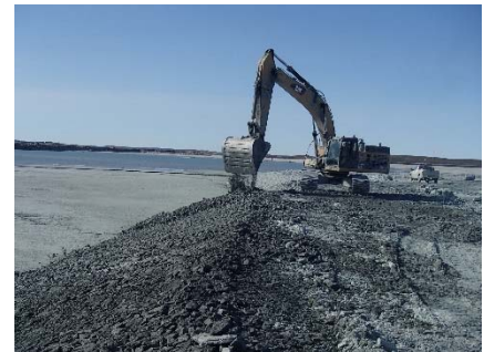
NCIS-063 (2018-06-30), looking SW from Sta. 1+200/-65 m. Placement of a 0.5 m thick lift of coarse filter in the upstream slope from El. 148 m to 150 m with an excavator from Sta. 1+270 m to 1+100 m.
