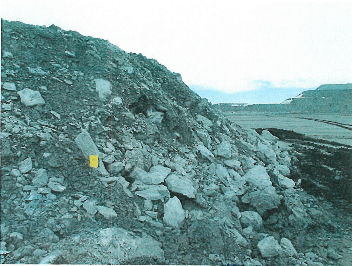
Photograph NCIS-028: From Sta. 1+340/+3 m, looking E. View of the LM rockfill lift approximately 3.2 m thick.
