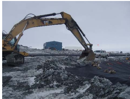
CD-1863 (2018-05-24), looking SW from Sta. 40+750/-18 m. Backfilling of the geosynthetic tie-in from Sta. 40+680 m to 0+950 m.
