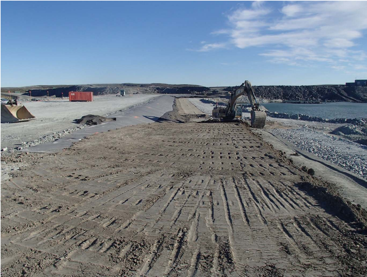
Photograph SD3-335: From Sta. 20+815/-27 m, looking N. Placement of a third 0.5 m thick lift of compacted sieved till on the upstream toe liner tie-in with an excavator from Sta. 20+760 m to 20+810 m.
