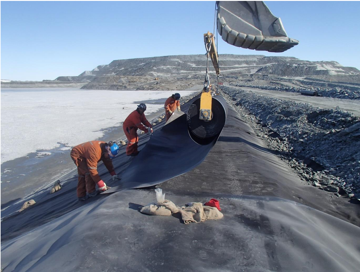
Photograph CD-1886: From Sta. 0+525/-26 m, looking N. Installation of the LLDPE liner on the upstream slope 2H:1V between El. 143 m and 145 m from Sta. 0+480 m to 0+320 m (panel numbers 887 to 910).
