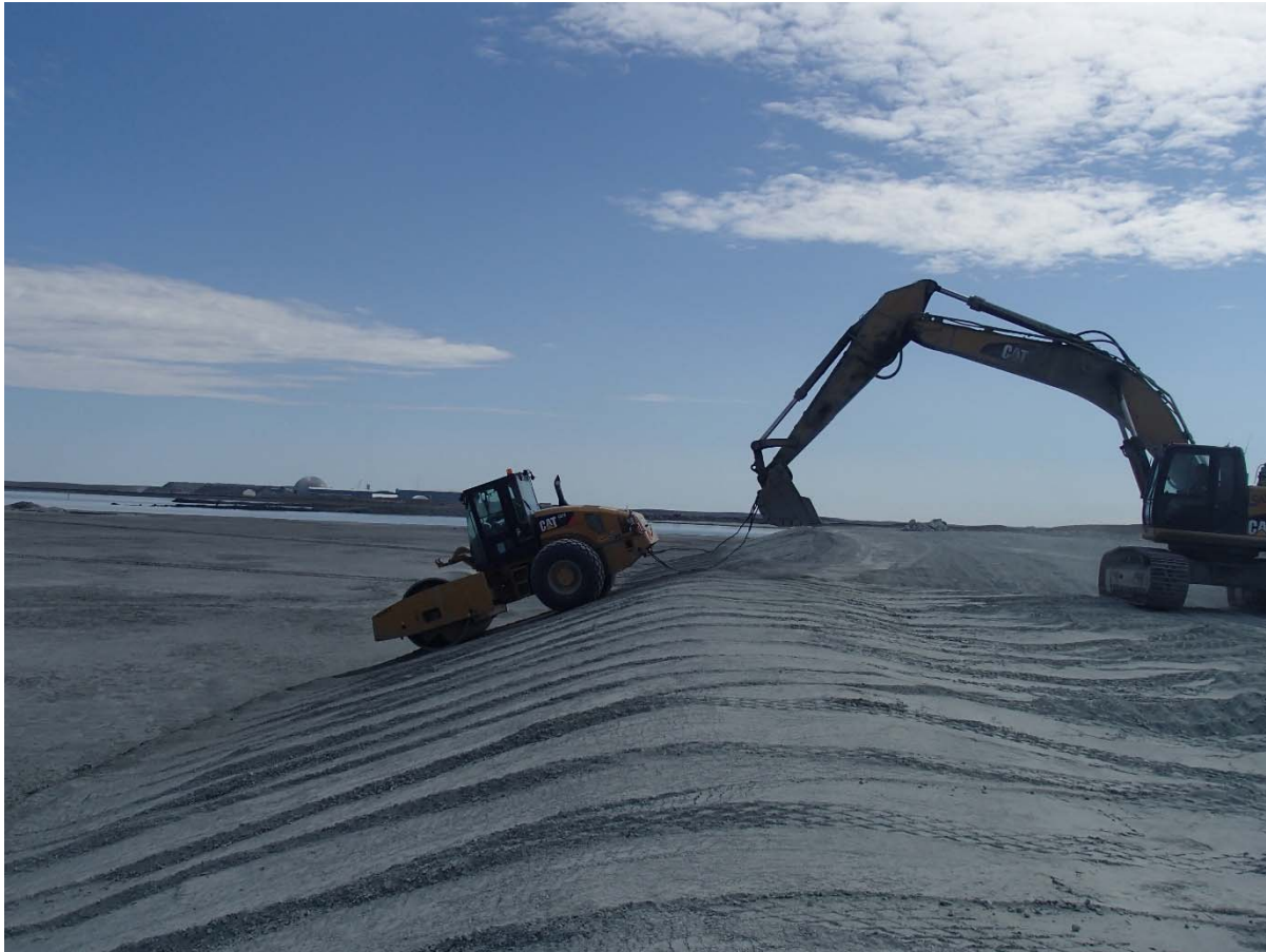
Photograph NCIS-107: From Sta. 1+380/-38 m (approx.), looking S. Compaction of the 0.5 m lift (approx.) of fine filter between El. 150 m and 152 m with a 10-tonne smooth-drum compactor with vibration (4 passes) in the upstream slope from Sta. 1+251 m to 1+660 m.
