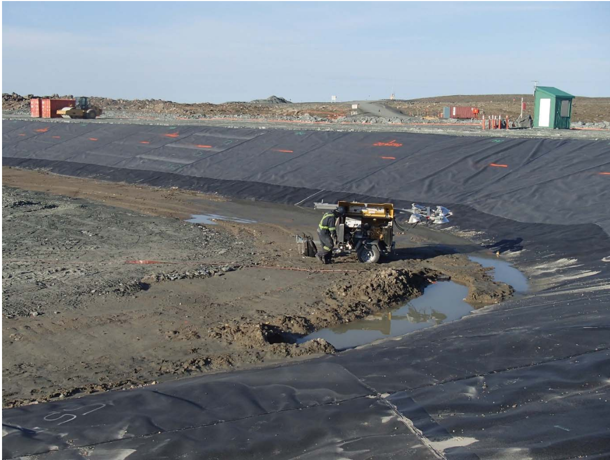
Photograph SD3-321: From Sta. 20+610/-56 m, looking SW. Water ponding at El. 142m on the compacted sieved till layer of the upstream toe liner tie-in at approx. Sta. 20+620 m to 20+630 m was pumped.
