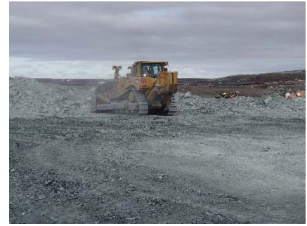
NCIS-048 (2018-06-26), looking SW from Sta. 1+120/-92 m. Placement of a 1.5 to 2 m thick (approx.) lift of UM rockfill from El. 148 m to El. 150 m (approx.) with a dozer from Sta. 1+125 m to 1+115 m (-92 m to -47 m).
