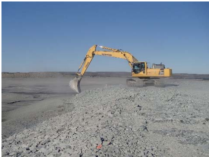
NCIS-094 (2018-07-15), looking SW from Sta. 1+125/-109 m (approx.). Profiling of the upstream slope (3H:1V) from El. 150 to 152 m with an excavator from Sta. 1+135 m to 1+115 m.
