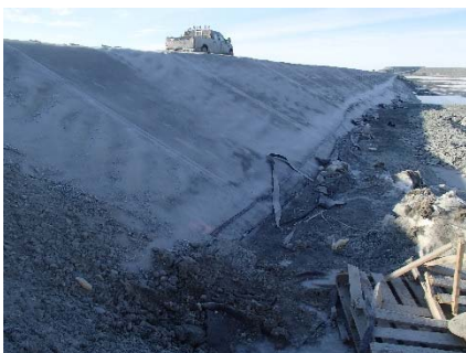
CD-1892 (2018-06-06), looking S from Sta. 0+155/-32 m. View of the liner panel 933 overlapping the underlying liner that has been cut at around Sta. 0+160 m to drain the water.
