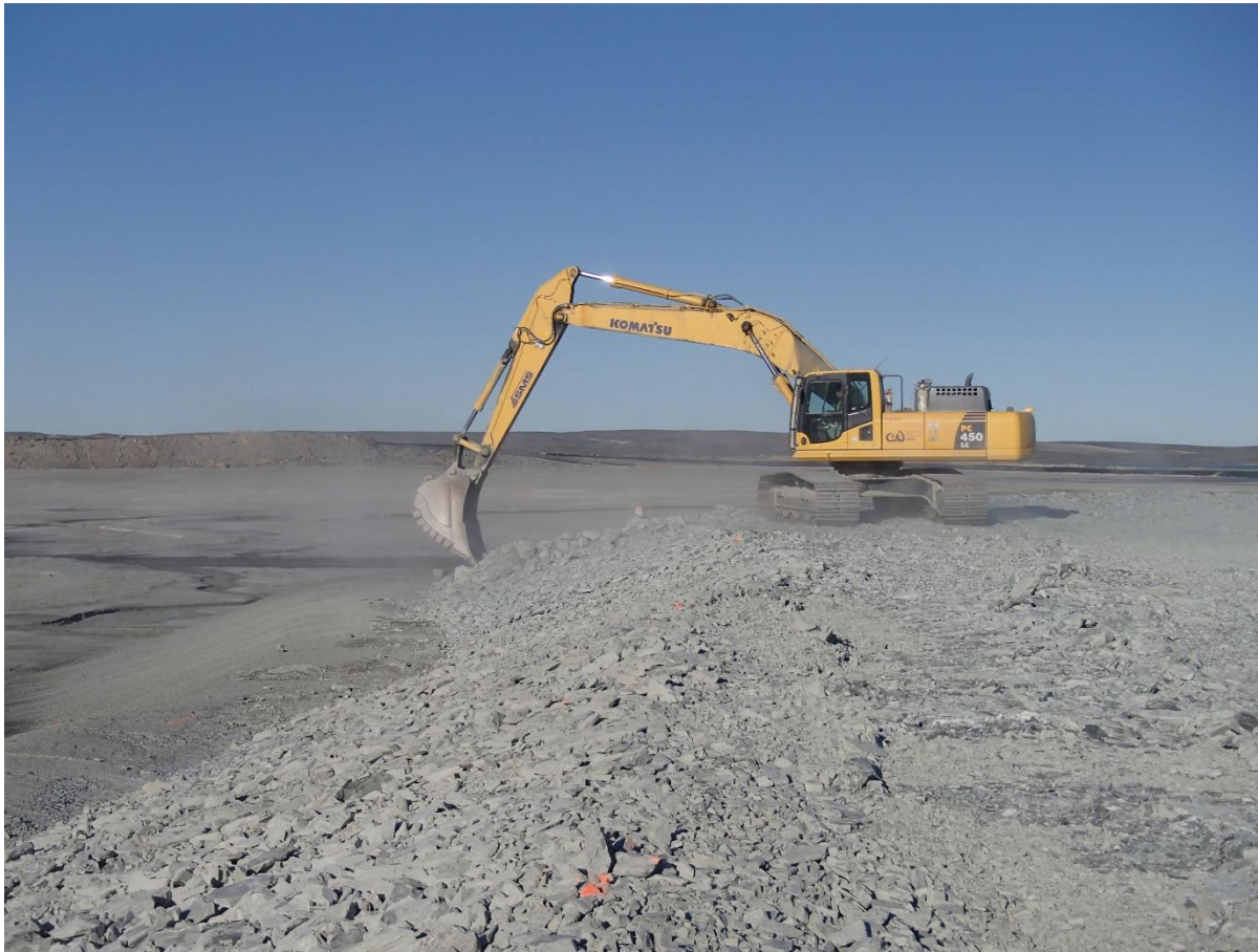
Photograph NCIS-094: From Sta 1+125/-109 m (approx.), looking SW. Profiling of the upstream slope (3H:1V) from El. 150 to 152 m with an excavator from Sta. 1+135 m to 1+100 m.
