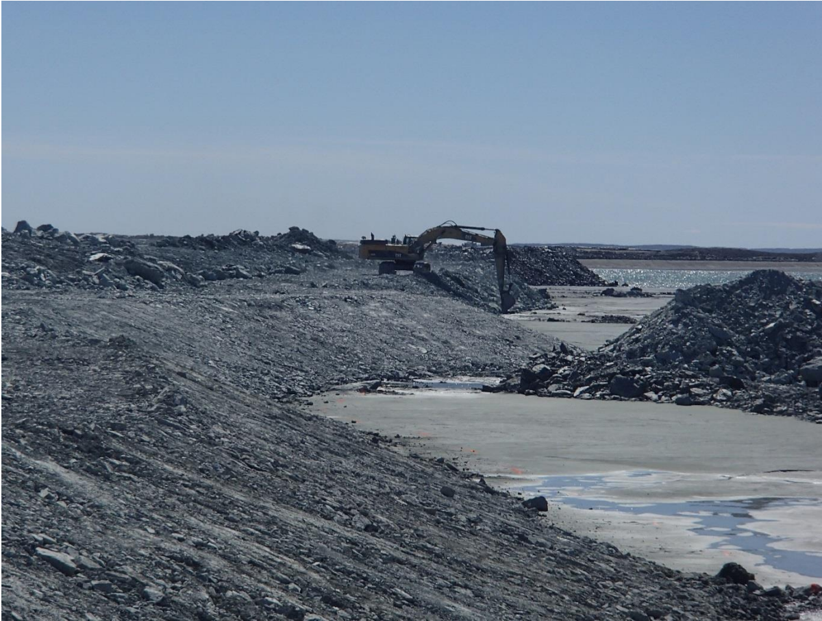
Photograph NCIS-072: From Sta. 2+790/-38 m (approx.), looking W. Profiling of the upstream slope (3H:1V) from El. 150 to 152 m with an excavator from Sta. 2+975 m to 3+070 m.
