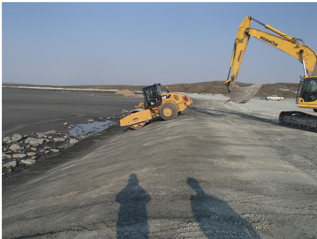
Photograph NCIS-088: From Sta 2+000/-35 m (approx.), looking W. Compaction of the 0.5 m lift (approx.) of fine filter between El. 150 m and 152 m with a 10-tonne smooth-drum compactor (4 passes) in the upstream slope from Sta. 2+028 m to 1+650 m.
