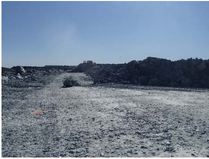
NCIS-100 (2018-07-20), looking E from Sta. 1+960/+10 m (approx.). Placement of a 2 m thick (approx.) lift of UM rockfill from El. 152 m to El. 154 m (approx.) with a dozer from Sta. 1+984 m to 1+947 m (+14 m to -26 m). The material is of good quality and is well graded.
