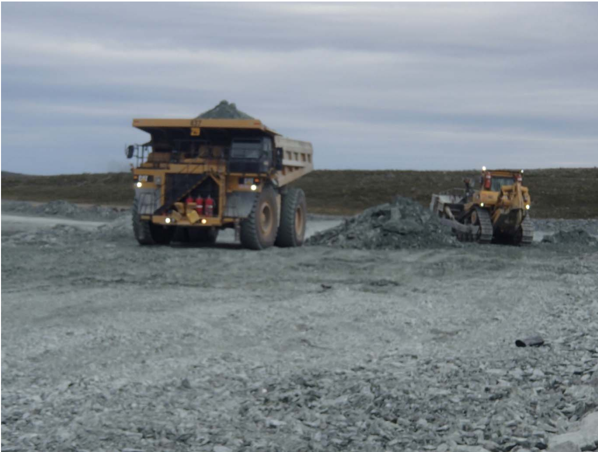
Photograph NCIS-096: From Sta 2+355/+9 m (approx.), looking N. Placement of a 2 m thick (approx.) lift of UM rockfill from El. 152 m to El. 154 m (approx.) with a dozer from Sta. 2+190 m to 2+103 m (+7 m to -22 m). The material is of good quality and is well graded.
