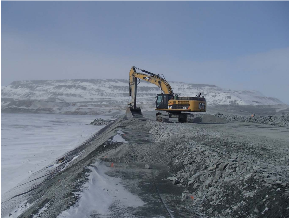
Photograph CD-1845: From Sta. 0+660/-20 m, looking N. Profiling of the upstream slope (2H:1V) from El. 143 to 145 m with an excavator between Sta. 0+175 and 0+330 m and between Sta. 0+600 m and 0+715 m. The removed material is placed on the fourth 0.5 m thick lift of fine filter from El. 144.5 m to 145 m upstream of the coarse filter with an excavator from Sta. 0+170 m to 0+330 m and between Sta. 0+600 m and 0+715 m.
