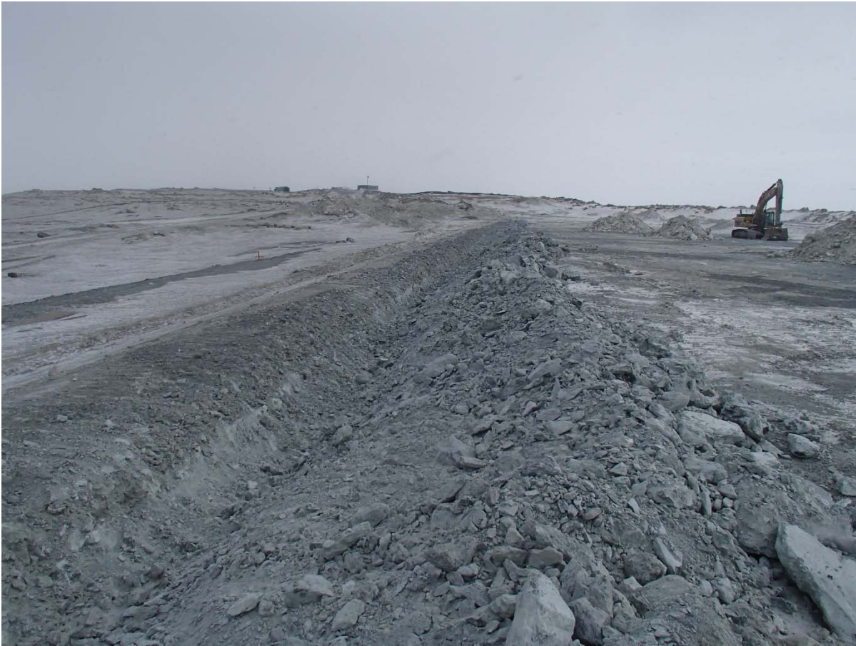
Photograph SD3-301: From Sta. 20+660/-22 m, looking SE. Excavation of the LLDPE geomembrane crest anchoring trench with an excavator from Sta. 20+655 m to 20+675 m.
