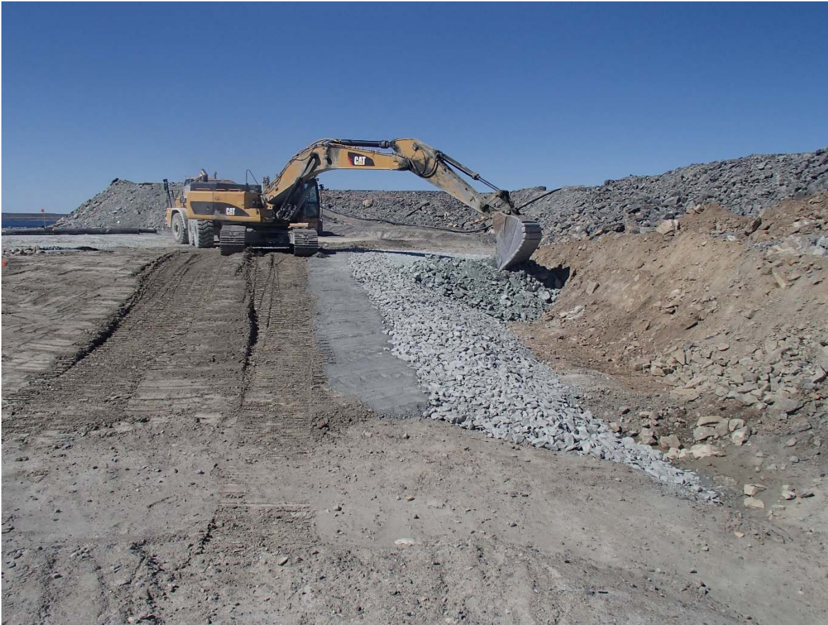
Photograph SD3-341: From Sta. 20+600/-58 m, looking W. Placement of a first 0.5 m thick lift of fine rockfill on the upstream slope of the upstream toe liner tie-in with an excavator from Sta. 20+588 m to 20+599 m.
