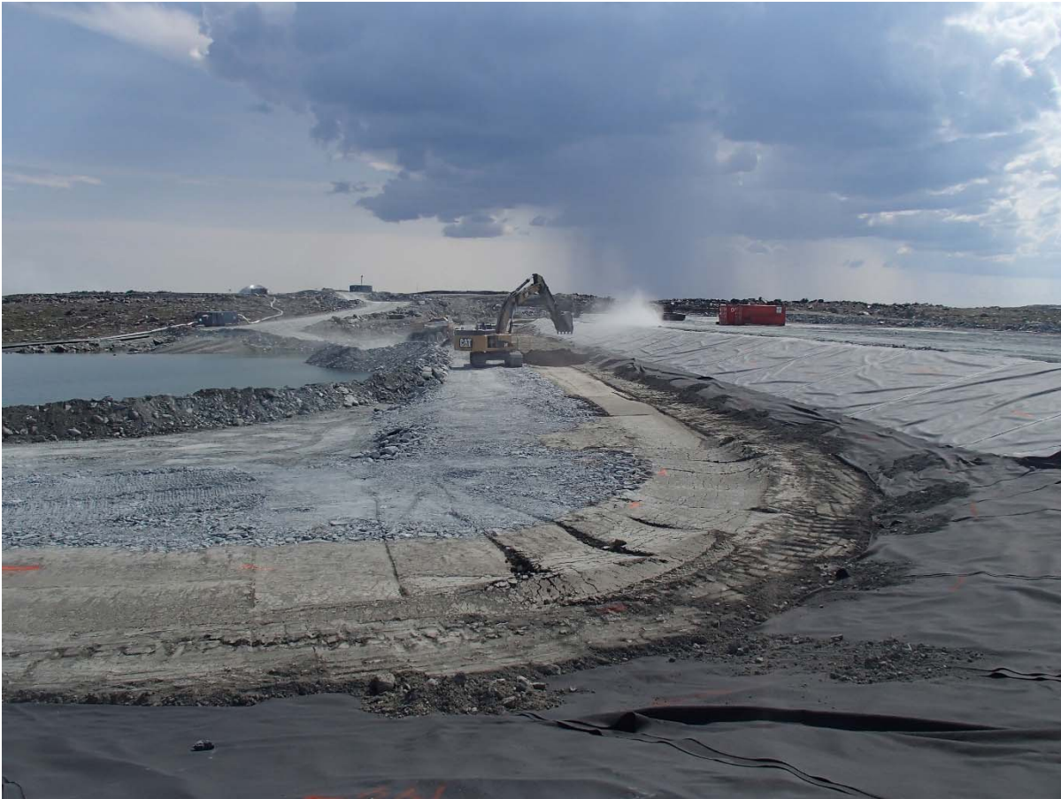
Photograph SD3-329: From Sta. 20+610/-43 m, looking S. Placement of a 0.5 m thick lift of low quality till (0-150 mm) from El. 142.5 m to 143 m from Sta. 20+610 m to 20+760 m.
