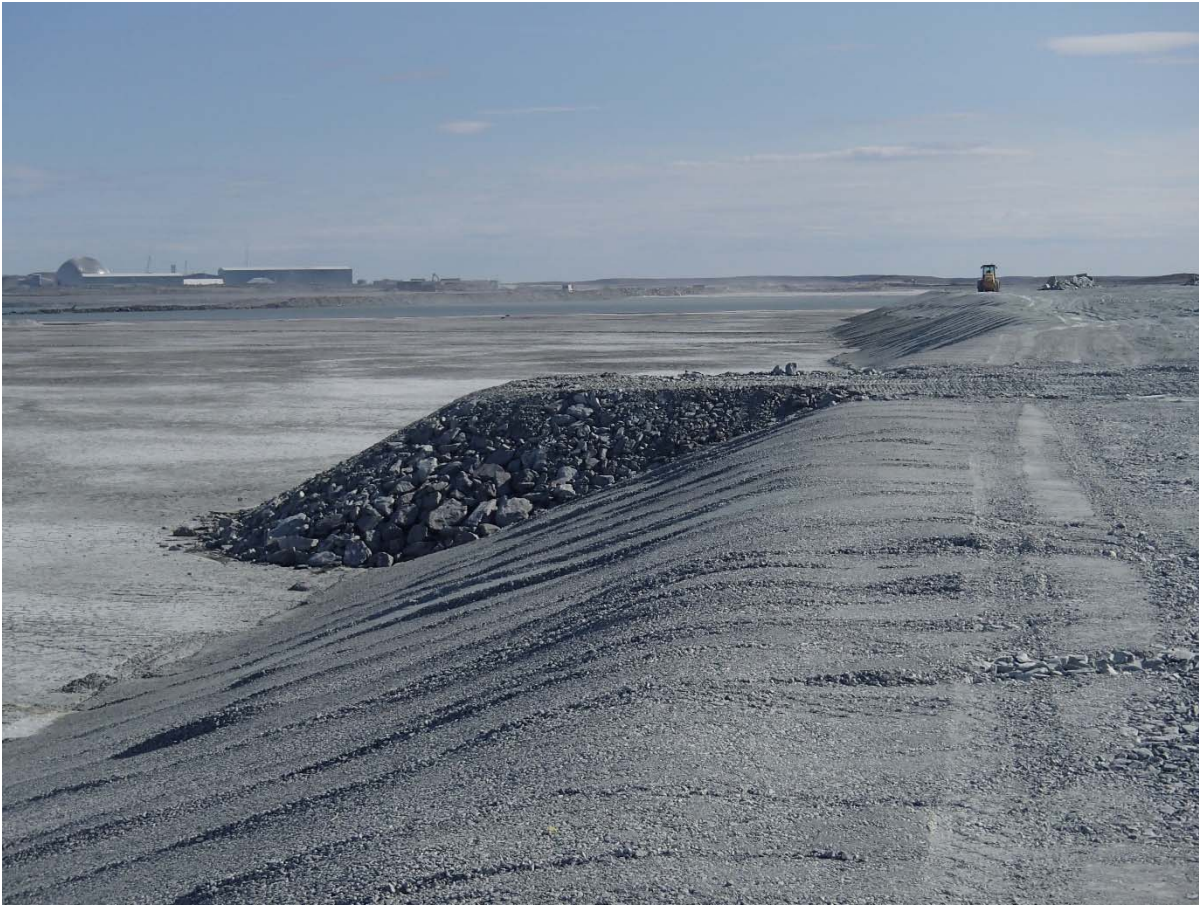
Photograph NCIS-118: From Sta. 1+500/-37 m (approx.), looking S. View of a deposition point.
