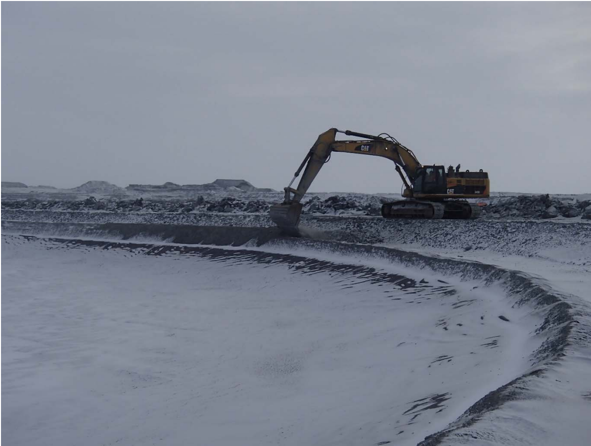
Photograph CD-1838: From Sta. 40+750/-31 m, looking NE. Placement of a second 0.5 m thick lift of fine filter from El. 143.5 m to 144 m upstream of the coarse filter with an excavator from Sta. 0+500 m to 0+835 m and from Sta. 0+930 to 40+730 m.
