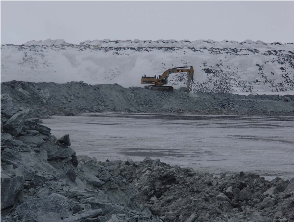
Photograph NCIS-012: From Sta. 2+000 m (approx.), looking NW. Profiling of the upstream slope (3H:1V) from El. 150 to 152 m with an excavator from Sta. 2+325 m to 2+275 m (approx.).
