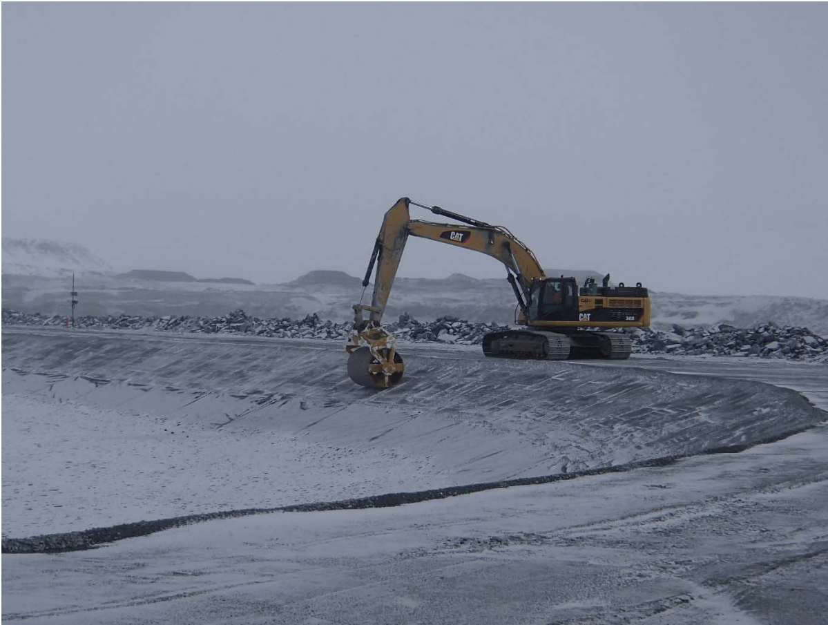
Photograph CD-1849: From Sta. 40+750/-17 m, looking NE. Final rolling of the upstream slope in view of the LLDPE geomembrane installation from Sta. 0+170 m to 40+730 m.
