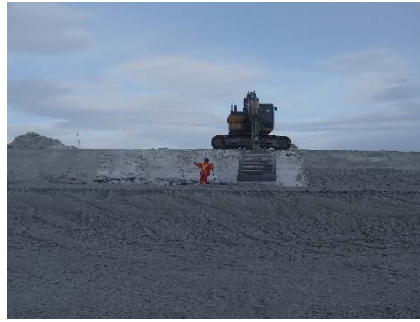
SD3-298 (2018-05-16), looking S from Sta. 20+680/-88 m. Removal of snow on the upstream slope of SD3 above El. 142 m, from Sta. 20+620 m to 20+780 m.
