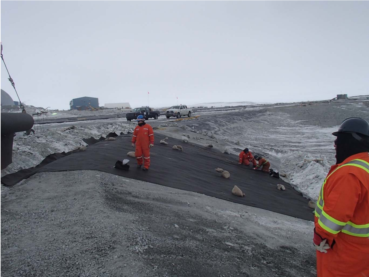
Photograph CD-1859: From Sta. 40+780/-38 m, looking SW. Installation of the geotextile on the upstream slope 3H:1V (SD5 side) to 2H:1V (Central Dike side) between El. 143 m and 145 m from Sta. 40+640 m to 0+830 m.
