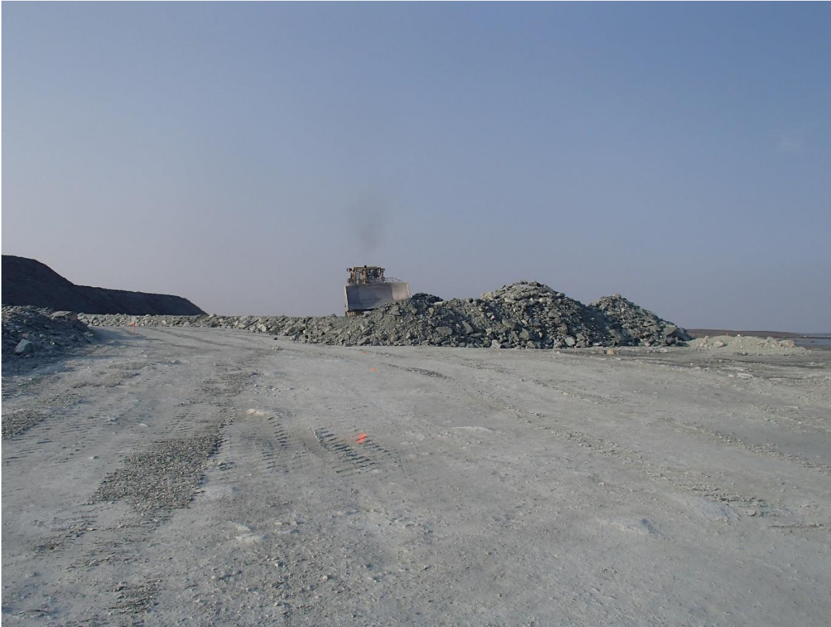
Photograph NCIS-089: From Sta 2+525/+4 m (approx.), looking S. Placement of a 2 m thick (approx.) lift of UM rockfill from El. 152 m to El. 154 m (approx.) with a dozer from Sta. 2+605 m to 2+455 m (+3 m to -23 m).
