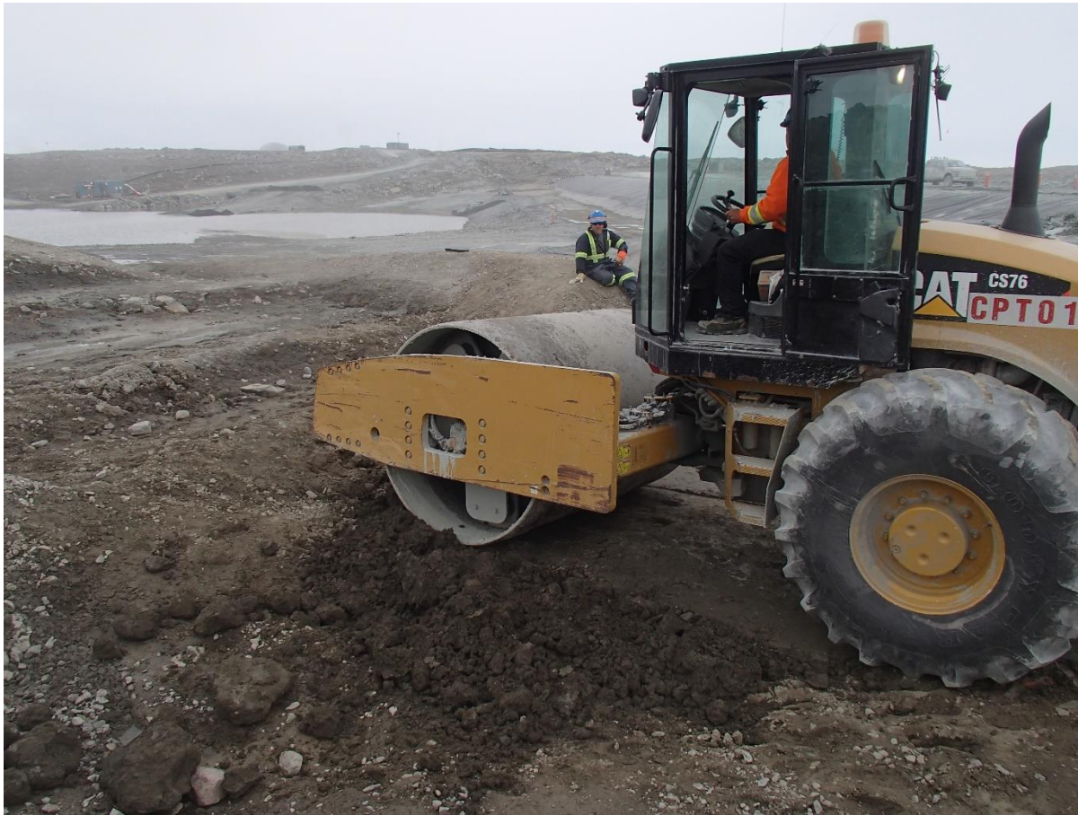
Photograph SD3-313: From Sta. 20+600/-52 m, looking S. Compaction of the 0.15 m-thick lift of compacted sieved till with a 10-tonne smooth-drum compactor without vibration from Sta. 20+596 m to 20+601 m.
