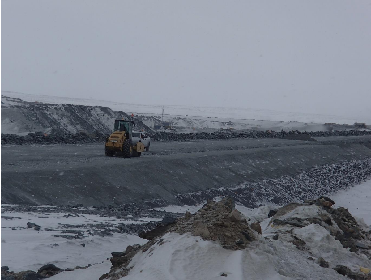
Photograph CD-1847: From Sta 0+085/-48 m, looking SE. Compaction of the fourth 0.5 m lift (approx.) of fine and coarse filters material at El. 145 m with a 10-tonne smooth-drum compactor with vibration (4 passes) from Sta 0+170 m to 0+930 m.
