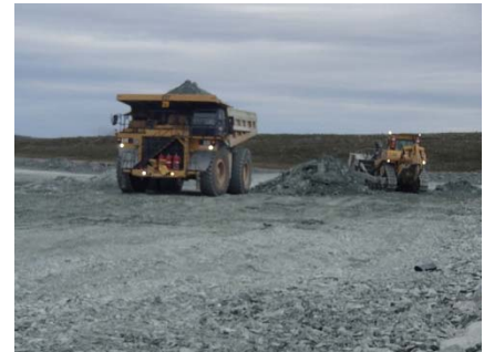
NCIS-096 (2018-07-18), looking N from Sta. 2+355/+9 m (approx.). Placement of a 2 m thick (approx.) lift of UM rockfill from El. 152 m to El. 154 m (approx.) with a dozer from Sta. 2+190 m to 2+103 m (+7 m to -22 m).
