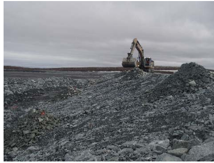
NCIS-047 (2018-06-26), looking N from Sta. 2+580/-35 m. Placement of a 0.5 m thick lift of coarse filter in the upstream slope from El. 150 m to 152 m with an excavator from Sta. 2+560 m to 2+640 m.
