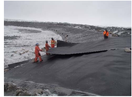
CD-1861 (2018-05-24), looking NE from Sta. 40+680/-8 m. Installation of the LLDPE liner on the upstream slope 3H:1V (SD5 side) to 2H:1V (Central Dike side) between El. 143 m and 145 m from Sta. 40+680 m to 0+950 m (panel numbers 802 to 817).
