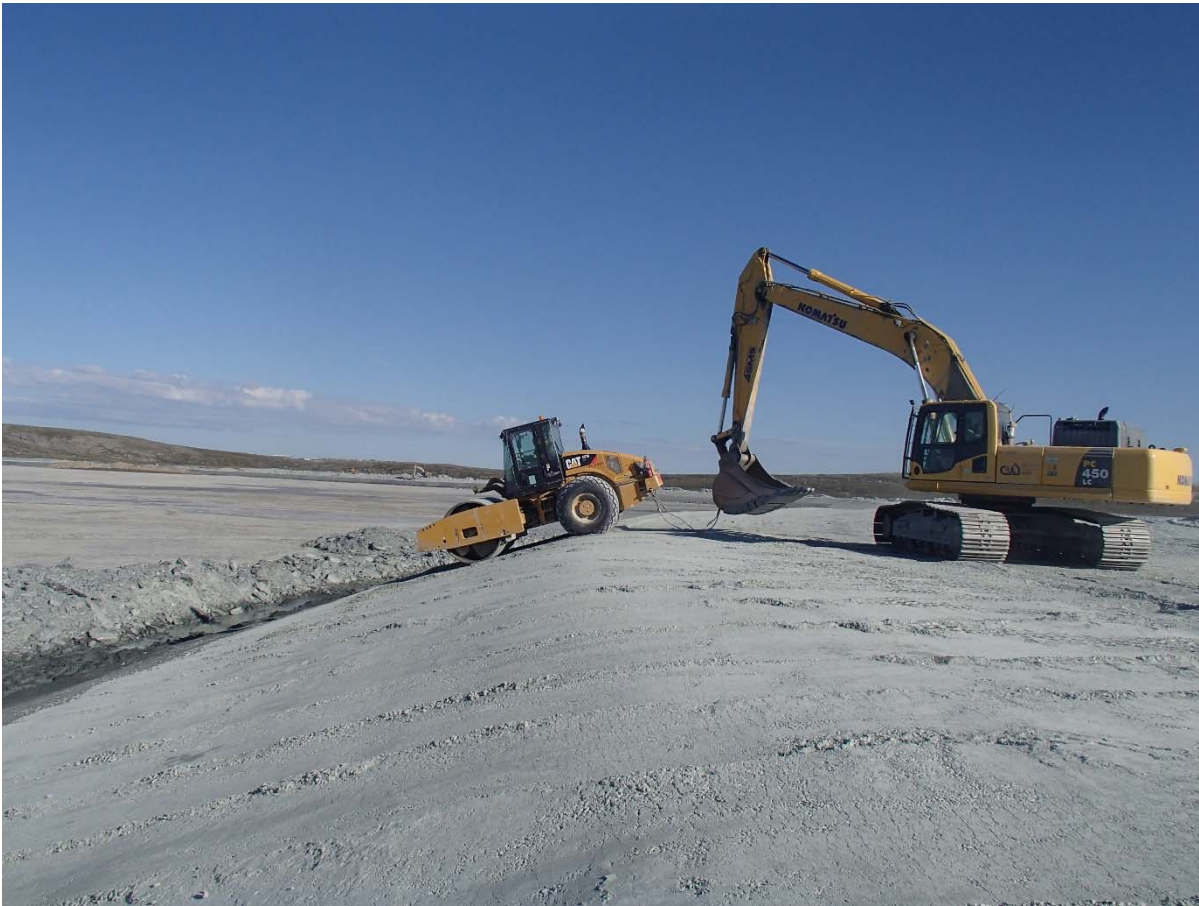
Photograph NCIS-112: From Sta. 2+610/-29 m (approx.), looking N. Compaction of the 0.5 m lift (approx.) of coarse filter between El. 152 m and 154 m with a 10-tonne smooth-drum compactor with vibration (4 passes) in the upstream slope from Sta. 2+080 m to 2+000 m.
