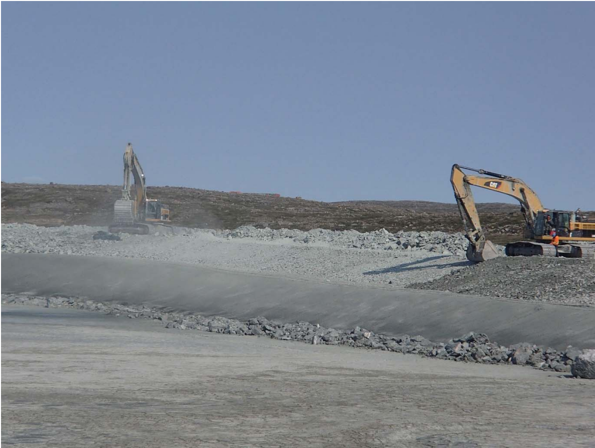
Photograph NCIS-111: From Sta. 2+320/-22 m (approx.), looking NW. Profiling of the upstream slope (3H:1V) from El. 152 to 154 m with an excavator from Sta. 2+159 m to 2+000 m and placement of a 0.5 m thick lift of coarse filter in the upstream slope from El. 152 m to 154 m with an excavator from Sta. 2+293 m to 2+080 m.
