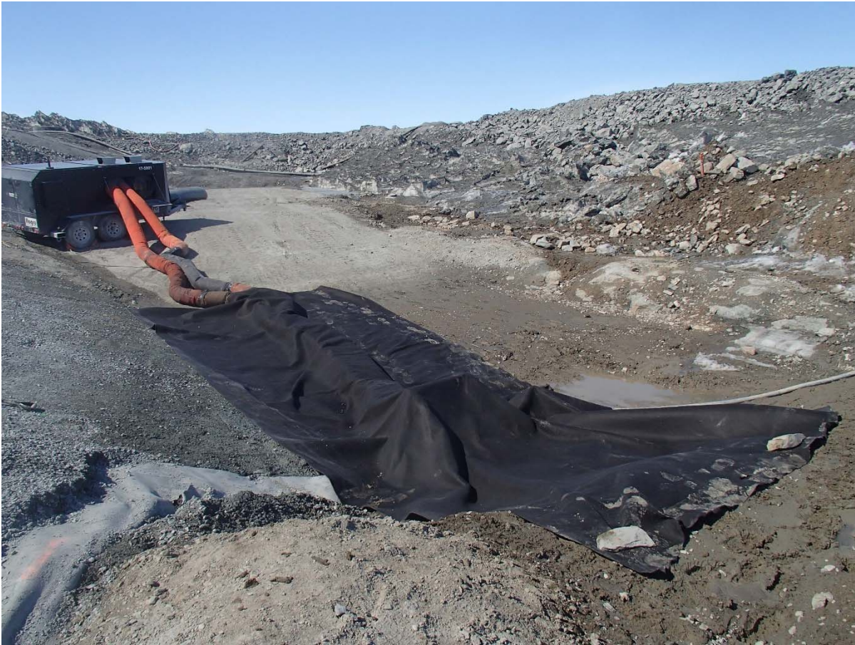
Photograph SD3-305: From Sta. 20+610/-48 m, looking NW. Dewatering of the water ponding on the first compacted sieved till layer of upstream toe liner tie-in. A Genset Frost-fighter is heating the sieved till layer and a pump is evacuating the water.
