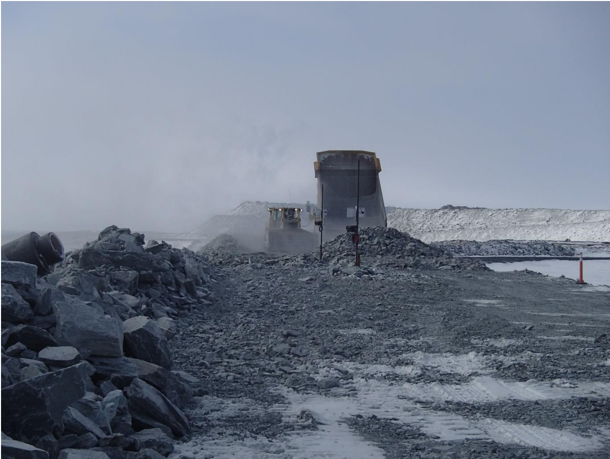
Photograph CD-1820: From Sta. 0+790/-7, looking S. Placement of a 2 m thick (approx.) lift of intermediate volcanic (IV) rockfill from El. 143 m to El. 145 m from approx. Sta. 0+880 m to 0+830 m (o.s. -28 to -11 m).
