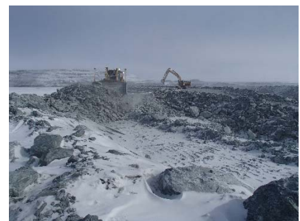
CD-1822 (2018-05-04), looking N from Sta. 40+725/+7 m. Placement of two 2 m thick lifts of IV rockfill from El. 141 m to El. 145 m from approx. Sta. 40+720 m to 40+750 m (o.s. -10 to +10 m) and profiling of the upstream slope (2H:1V) from El. 143 to 145 m with an excavator between Sta. 0+830 m and 0+980 m.
