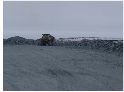
NCIS-021 (2018-05-28), looking S from Sta. 1+550 m. Placement a 2 m thick (approx.) lift of UM rockfill from El. 150 m to El. 152 m (approx.) with a dozer from Sta. 1+535 m to 1+500 m (o.s. unavailable).
