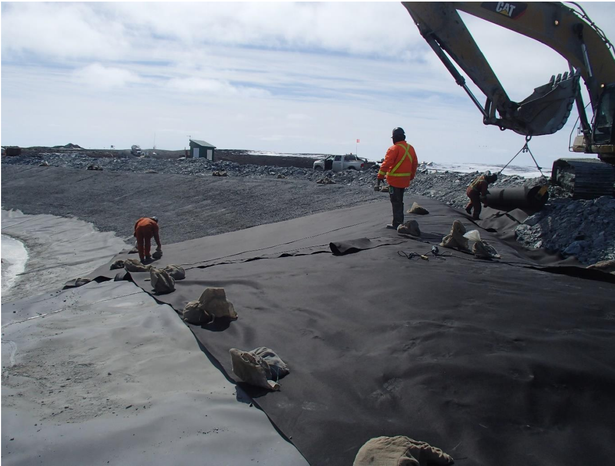
Photograph SD-308: From Sta. 20+620/-48 m, looking SW. Installation of the geotextile on the upstream slope 2H:1V between El. 143 m and 145 m from Sta. 20+620 m to 20+630 m.
