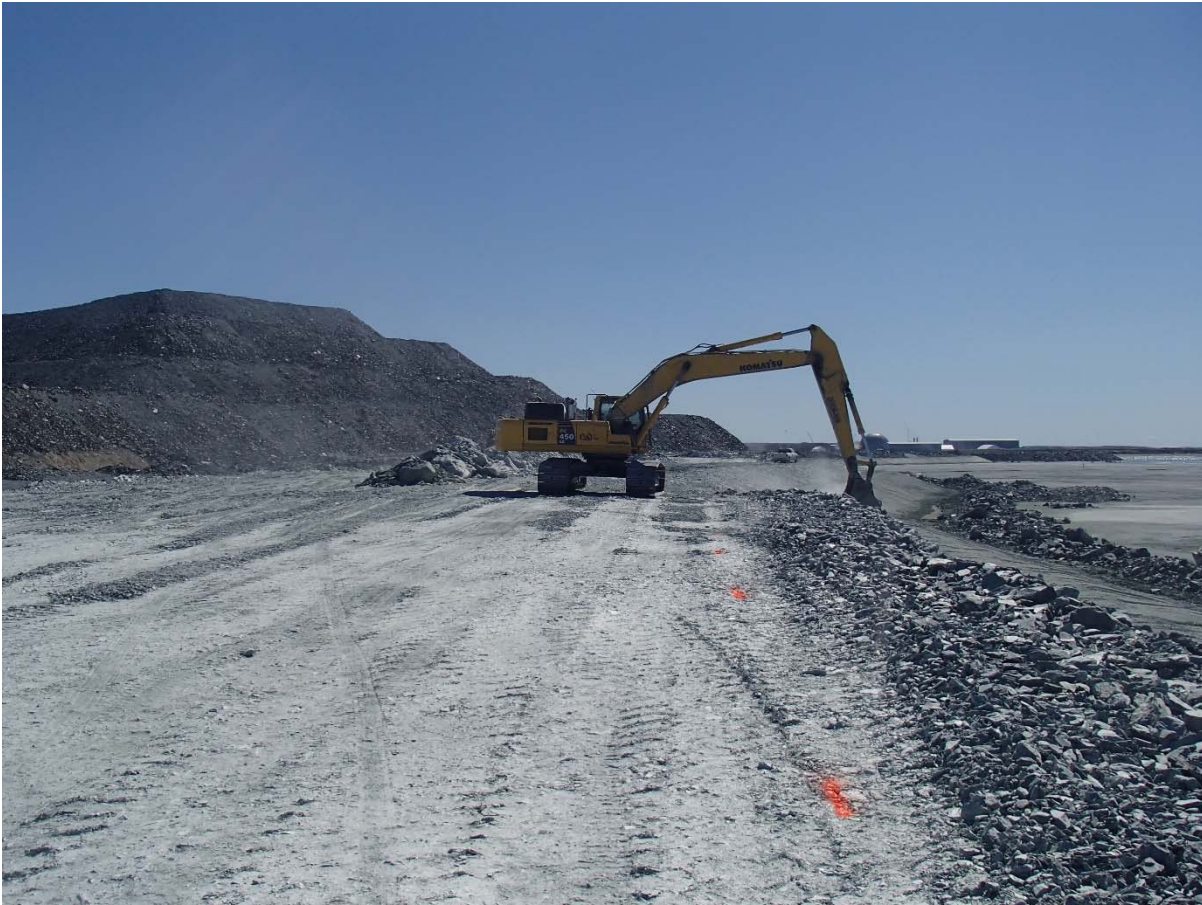
Photograph NCIS-095: From Sta 2+375/-18 m (approx.), looking S. Profiling of the upstream slope (3H:1V) from El. 152 to 154 m with an excavator from Sta. 2+545 m to 2+410 m.
