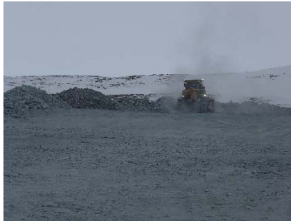
NCIS-011 (2018-05-22), looking SW from Sta. 2+000 m. Placement a 2 m thick (approx.) lift of UM rockfill from El. 150 m to El. 152 m (approx.) with a dozer from Sta. 1+880 m to 1+767 m (o.s. unavailable).
