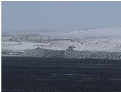
NCIS-023 (2018-05-31), looking W from Sta. 2+570 m. Placement of a 2 m thick (approx.) lift of UM rockfill from El. 150 m to El. 152 m (approx.) with a dozer from Sta. 1+500 m to 1+450 m (o.s. unavailable). The material is of good quality and is well graded.
