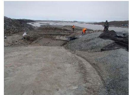
SD3-314 (2018-06-08), looking E from Sta. 20+590/-32 m. View of the liner bedding ready for geosynthetics installation.
