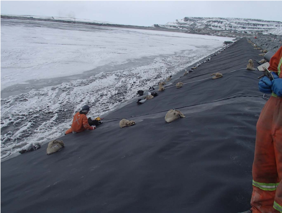
Photograph CD-1866: From Sta. 0+940/-25 m, looking NW. Installation of the LLDPE liner on the upstream slope 2H:1V between El. 143 m and 145 m from Sta. 0+950 m to 0+935 m (panel numbers 818 and 819).
