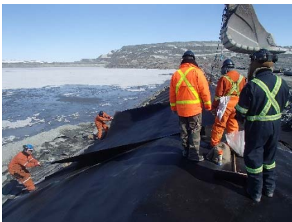
CD-1883 (2018-06-02), looking N from Sta. 0+525/-26 m. Installation of the LLDPE liner on the upstream slope 2H:1V between El. 143 m and 145 m from Sta. 0+610 m to 0+480 m (panel numbers 868 to 886).
