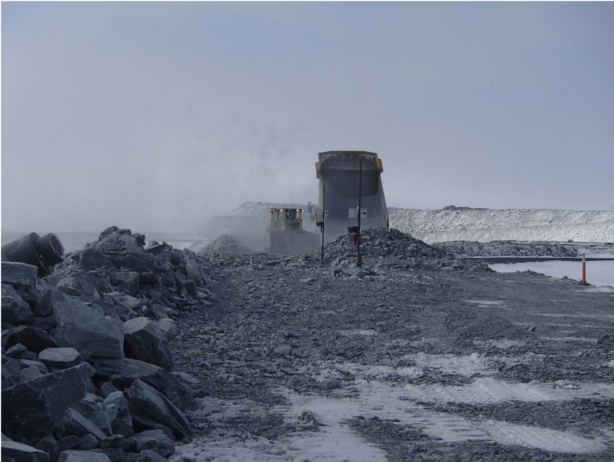
Photograph CD-1820: From Sta. 0+790/-7, looking S. Placement of a 2 m thick (approx.) lift of intermediate volcanic (IV) rockfill from El. 143 m to El. 145 m from approx. Sta. 0+880 m to 0+830 m (o.s. -28 to -11 m).
