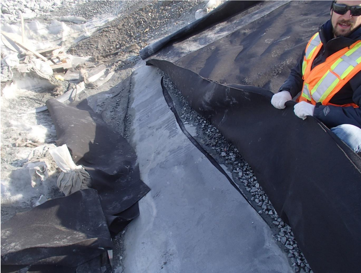
Photograph CD-1889: From Sta. 0+150/-28 m, looking N. View of the underlying liner that has been cut at around Sta. 0+160 m to drain the water.
