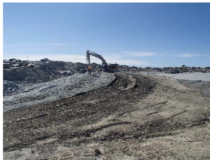
SD3-336 (2018-07-14), looking S from Sta. 20+755/-48 m. Placement of a fourth 0.5 m thick lifts of fine filter, coarse filter and fine rockfill on the upstream slope of the upstream toe liner tie-in with an excavator from Sta. 20+770 to 20+800 m.
