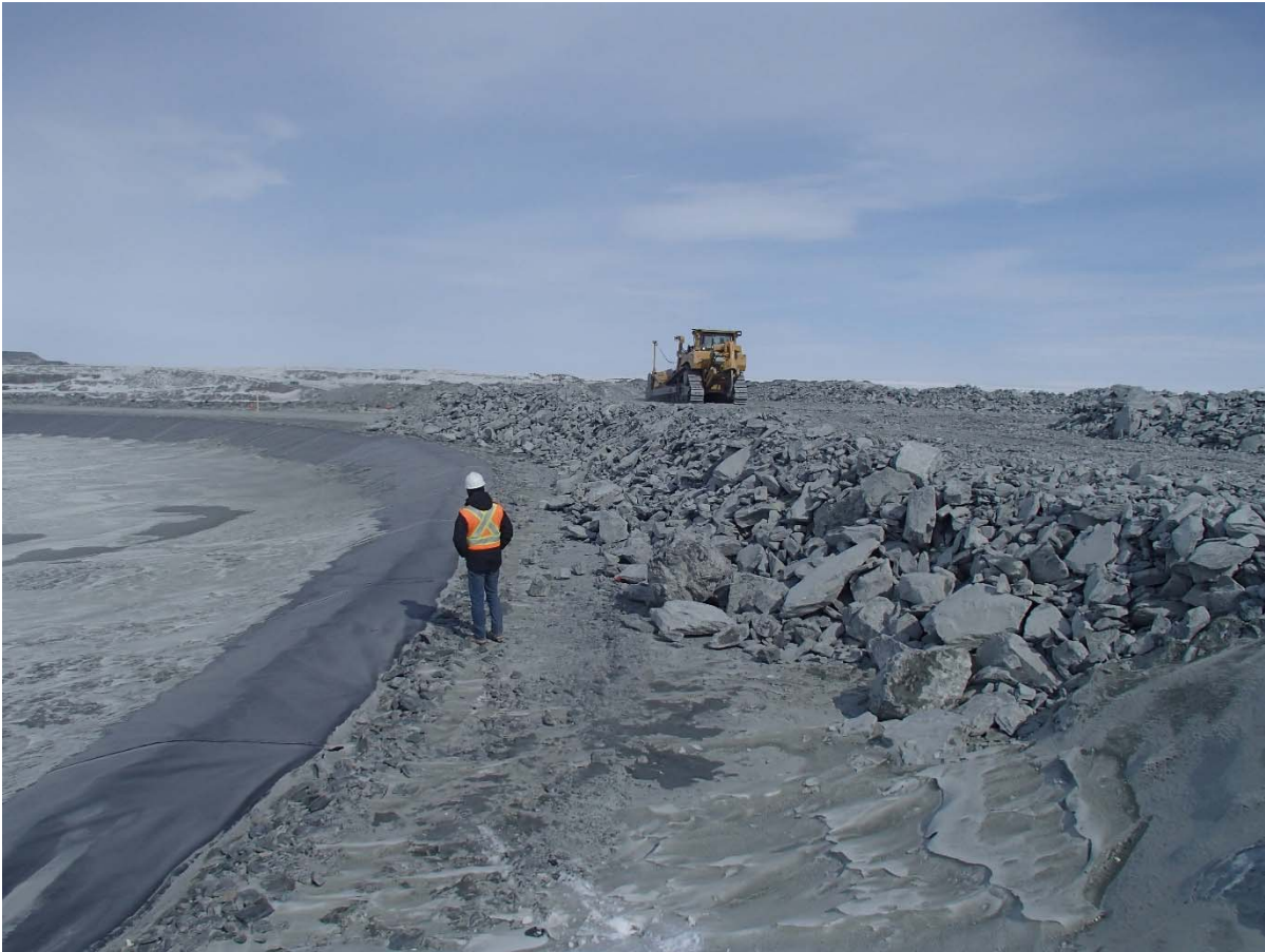
Photograph CD-1817: From Sta. 40+700/-10, looking NE. View of the rockfill lift thickness at the junction of Saddle Dam 5 and Central Dike, approx. 2.5 m thick.
