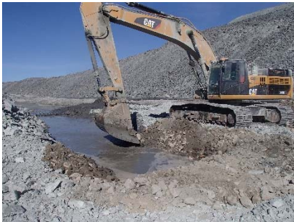
NCIS-121 (2018-07-26), looking NE from Sta. 3+050/+26 m (approx.). Placement of a 0.3 m thick (approx.) layer of till sieving reject material on the bottom and on the slopes of the sump.
