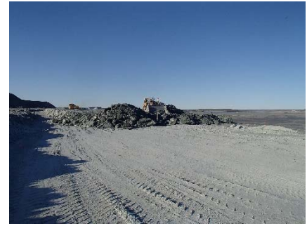
NCIS-093 (2018-07-15), looking S from Sta. 2+260/+12 m (approx.). Placement of a 2 m thick (approx.) lift of UM rockfill from El. 152 m to El. 154 m (approx.) with a dozer from Sta. 2+290 m to 2+280 m (+9 m to -22 m).
