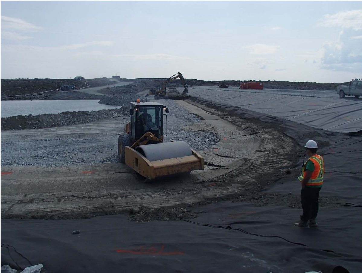
Photograph SD3-328: From Sta. 20+610/-43 m, looking S. Compaction perpendicularly to the longitudinal axe of Saddle Dam 3 of the 0.5 m lift of low quality till (0-150 mm) at El. 142.5 m with a 10-tonne smooth-drum compactor without vibration (4 passes) from Sta. 20+615m to 20+635 m.
