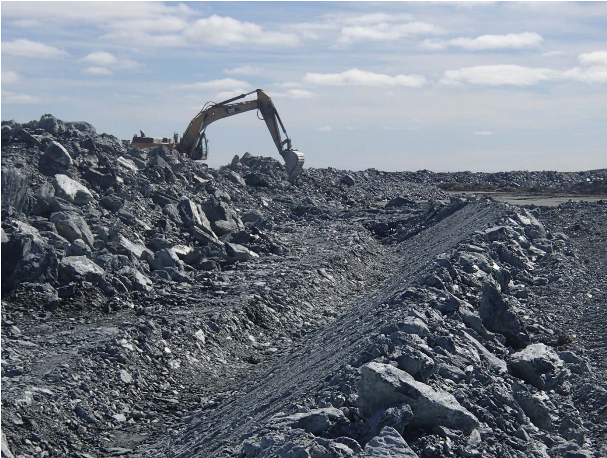
Photograph NCIS-130: From Sta. 1+446/+16 m (approx.), looking S. Excavation of a 0.8 m (approx.) deep, 1 m wide shallow ditch in the rockfill capping with an excavator from Sta. 1+380 m to 1+300 m.
