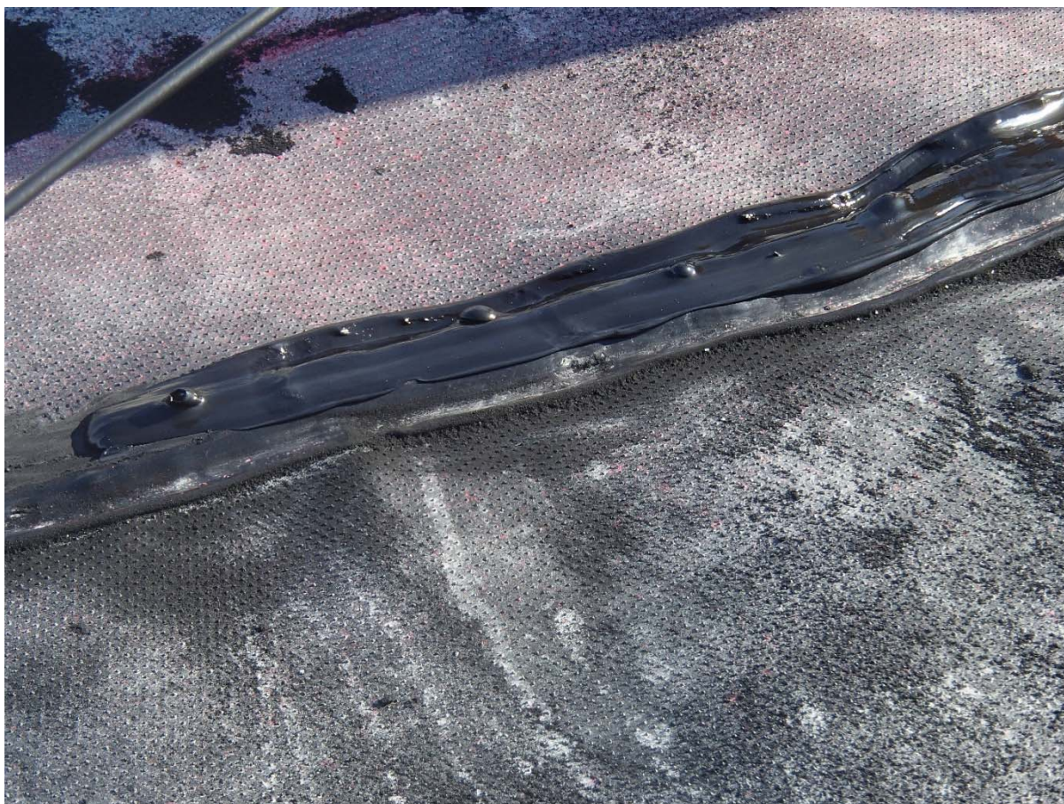
Photograph CD-1864: From Sta. 40+700/-38 m. View of bubbles formed in the extrusion weld because of humidity.
