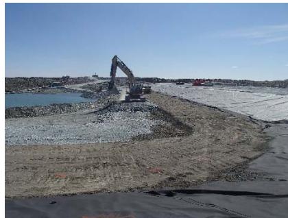
SD3-330 (2018-07-12), looking S from Sta. 20+610/-43 m. Placement of a second 0.5 m thick lift of fine rockfill (0-500 mm) upstream of the low quality till (0-150mm) from El. 142.5 m to 143 m from Sta. 20+610 m to 20+760 m.
