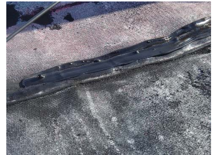
CD-1864 (2018-05-25), looking from Sta. 40+700/-38 m. View of bubbles formed in the extrusion weld because of humidity.
