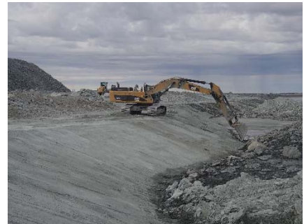
NCIS-078 (2018-07-05), looking S from Sta. 2+760/-39 m. Placement of a 0.5 m thick lift of fine filter over the coarse filter in the upstream slope from El. 150 m to 152 m with an excavator from Sta. 2+800 m to 2+980 m.
