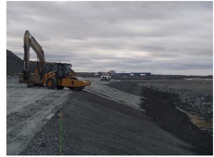
NCIS-129 (2018-07-28), looking S from Sta. 2+450/-21 m (approx.). Compaction of the 0.5 m lift (approx.) of fine filter between El. 152 m and 154 m with a 10-tonne smooth-drum compactor with vibration (4 passes) in the upstream slope from Sta. 2+220 m to 1+940 m.
