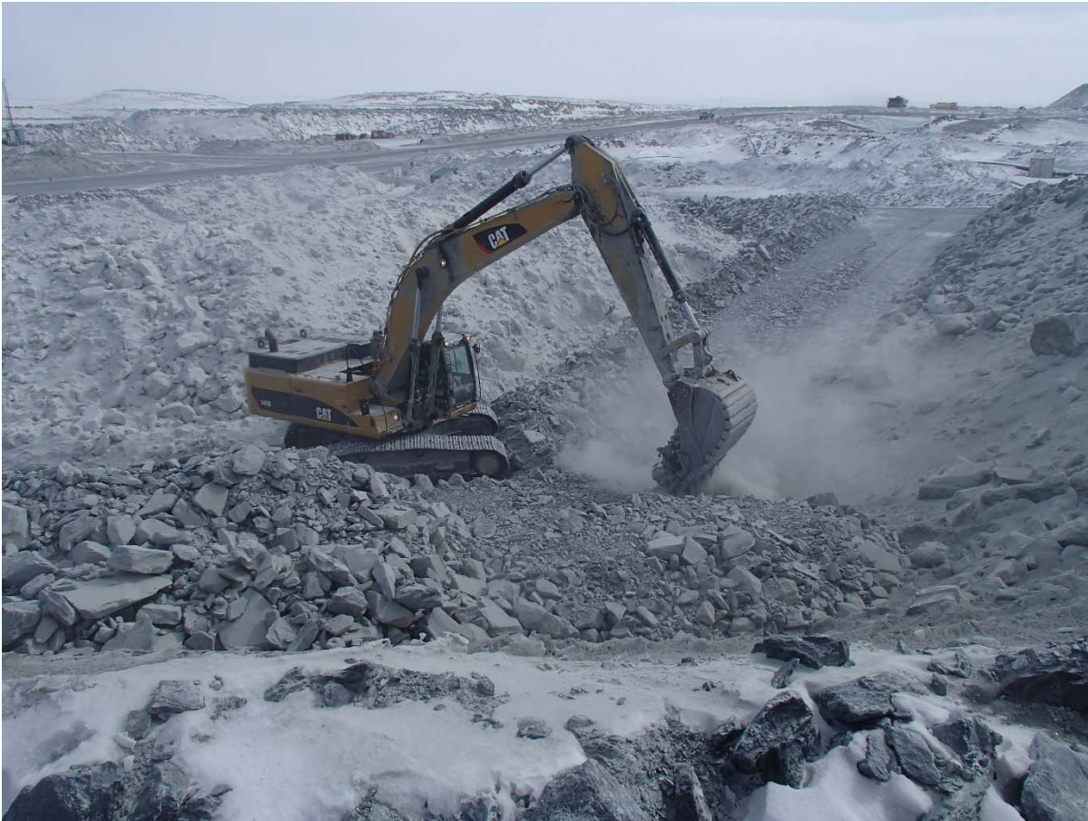
Photograph CD-1812: From Sta. 0+985/-11 m looking SE. Placement of intermediate volcanic (IV) rockfill on the existing downstream slope up to approx. El. 140 m, from approx. Sta. 0+985 to 40+780 m.
