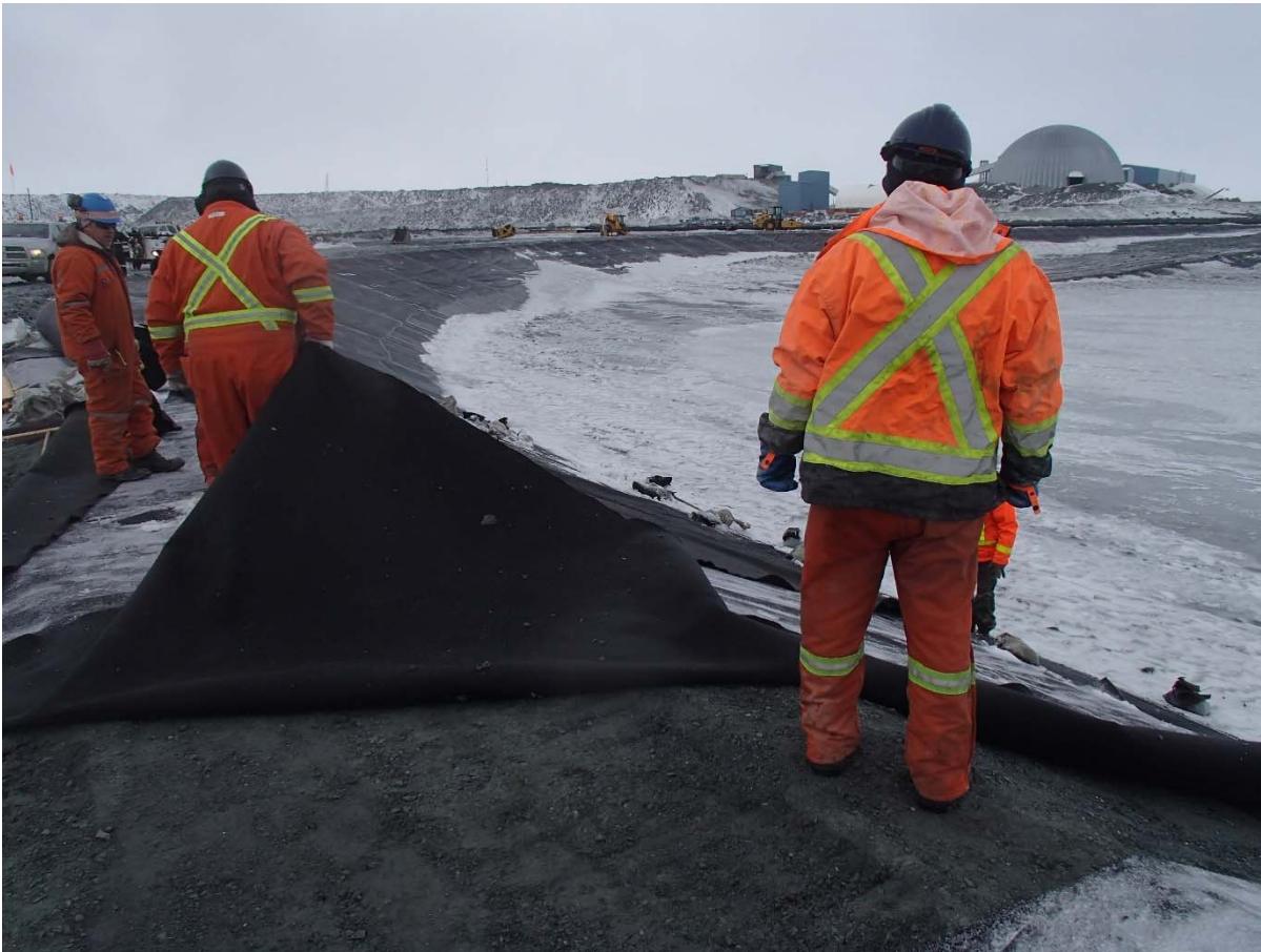
Photograph CD-1868: From Sta. 0+915/-24 m, looking S. Removal of the wet geotextile in place from Sta. 0+935 m to 0+900 m.
