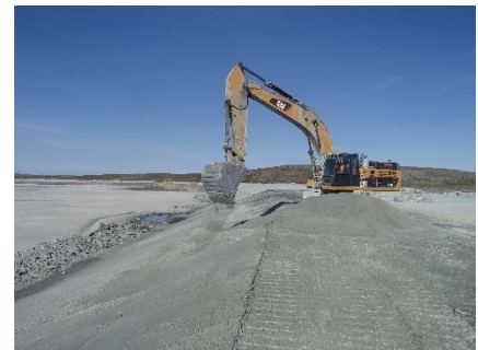
NCIS-117 (2018-07-25), looking SW from Sta. 2+050/-25 m (approx.). Placement of a 0.5 m thick lift of fine filter in the upstream slope from El. 152 m to 154 m with an excavator from Sta. 2+090 m to 1+890 m.
