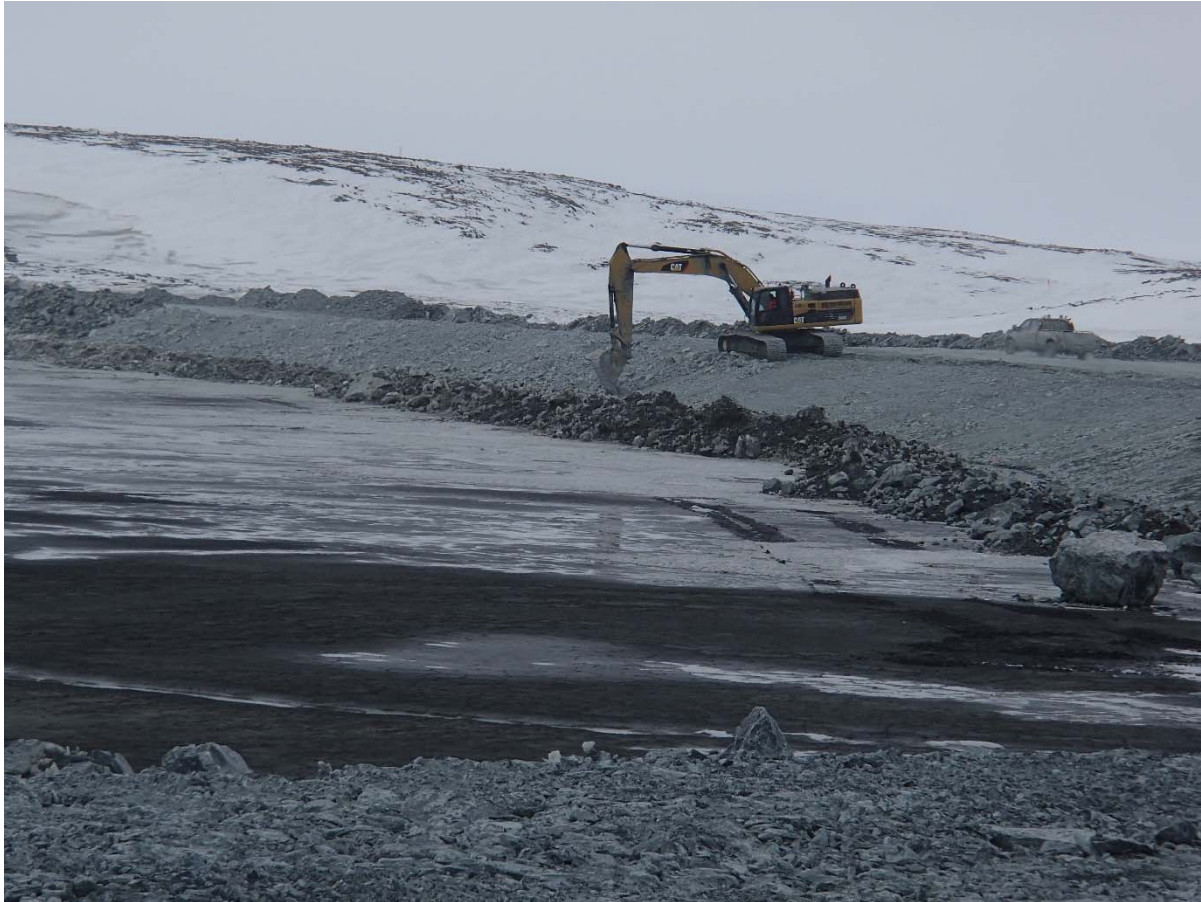
Photograph NCIS-017: From Sta. 2+290 m (approx.), looking SW. Profiling of the upstream slope (3H:1V) from El. 150 to 152 m with an excavator from Sta. 2+138 m to 1+989 m.
