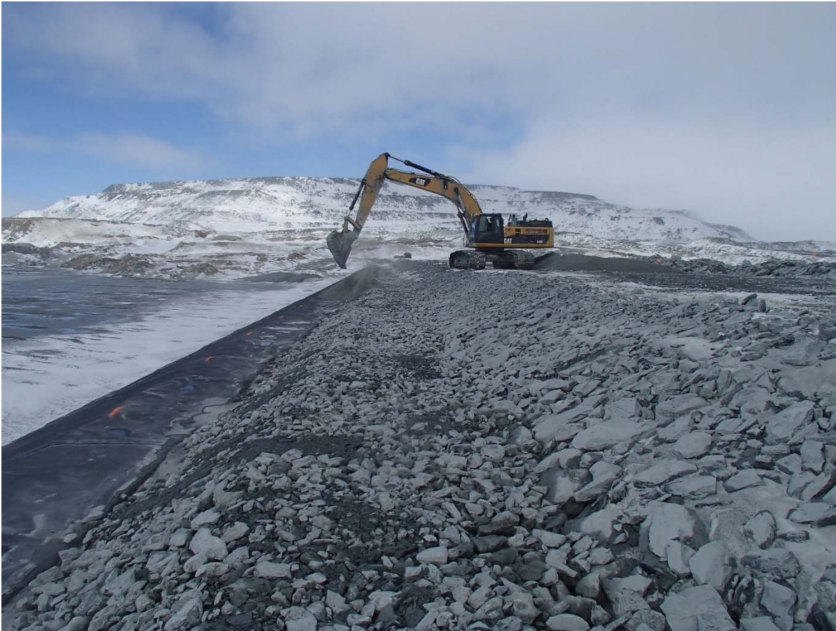
Photograph CD-1829: From Sta 0+410/-22 m, looking N. Placement of a 0.5 m thick lift of coarse filter from El. 143 m to 143.5 m with an excavator from Sta. 0+170 m to 0+460 m and placement of a 0.5 m thick lift of fine filter from Sta. 0+170 m to 0+380 m.
