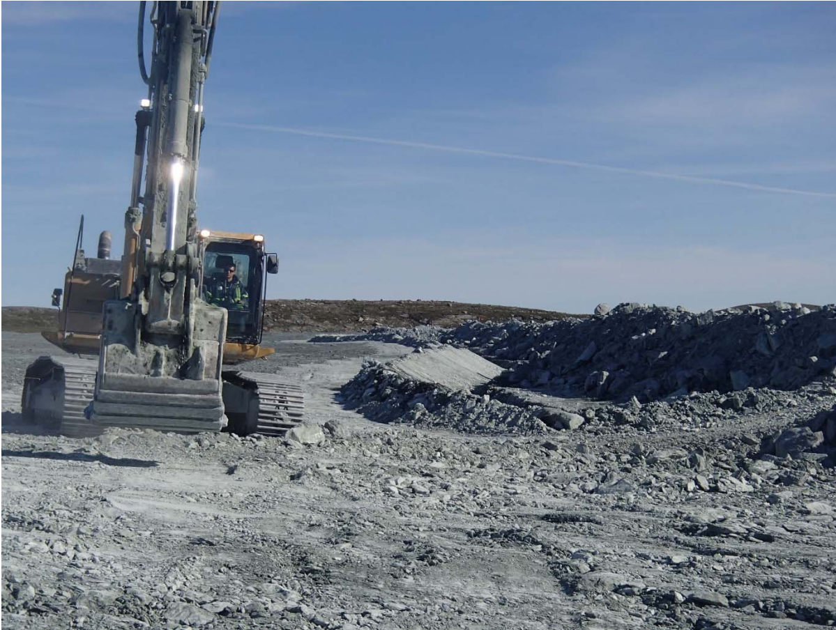
Photograph NCIS-119: From Sta. 1+430/-22 m (approx.), looking N. Excavation of a 0.8 m (approx.) deep, 1 m wide shallow ditch in the rockfill capping with an excavator from Sta. 1+455 m to 1+400 m.
