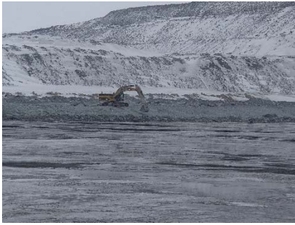
NCIS-010 (2018-05-21). Profiling of the upstream slope (3H:1V) from El. 150 to 152 m with an excavator from Sta. 2+777 m to 2+400 m.
