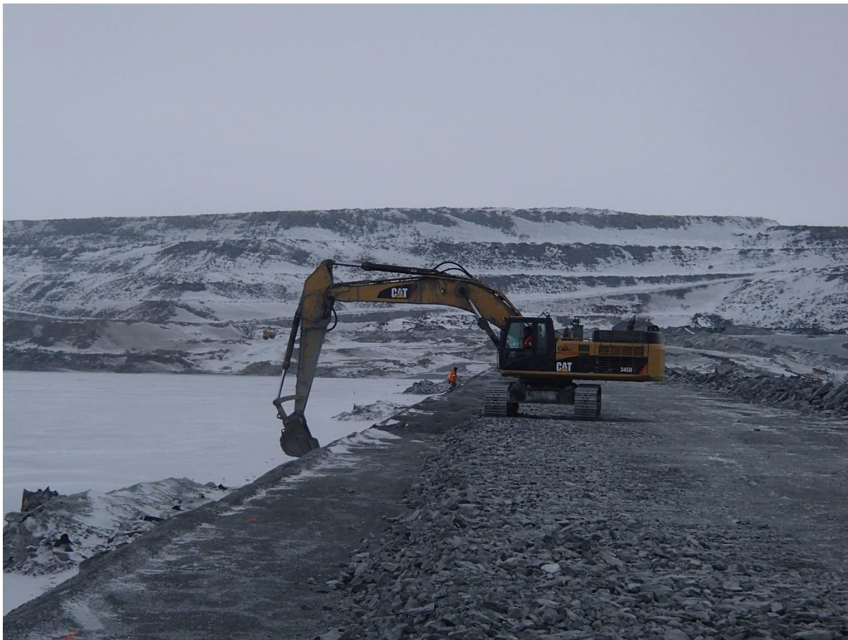
Photograph CD-1846: From Sta 0+835/-25 m, looking N. Profiling of the upstream slope (2H:1V) from El. 143 to 145 m with an excavator between Sta. 0+330 and 0+600 m and between Sta. 0+715 m and 40+730 m. The removed material was placed with material from the fine filter stockpile on the fourth 0.5 m thick lift of fine filter from El. 144.5 m to 145 m upstream of the coarse filter with an excavator from Sta. 0+330 m to 0+600 m and between Sta. 0+715 m and 40+730 m.
