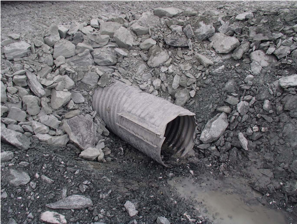
Photograph NCIS-127: From Sta. 1+470/+20 m (approx.), looking SW. View of the culvert installed in the ditch at Sta. 1+460 m.
