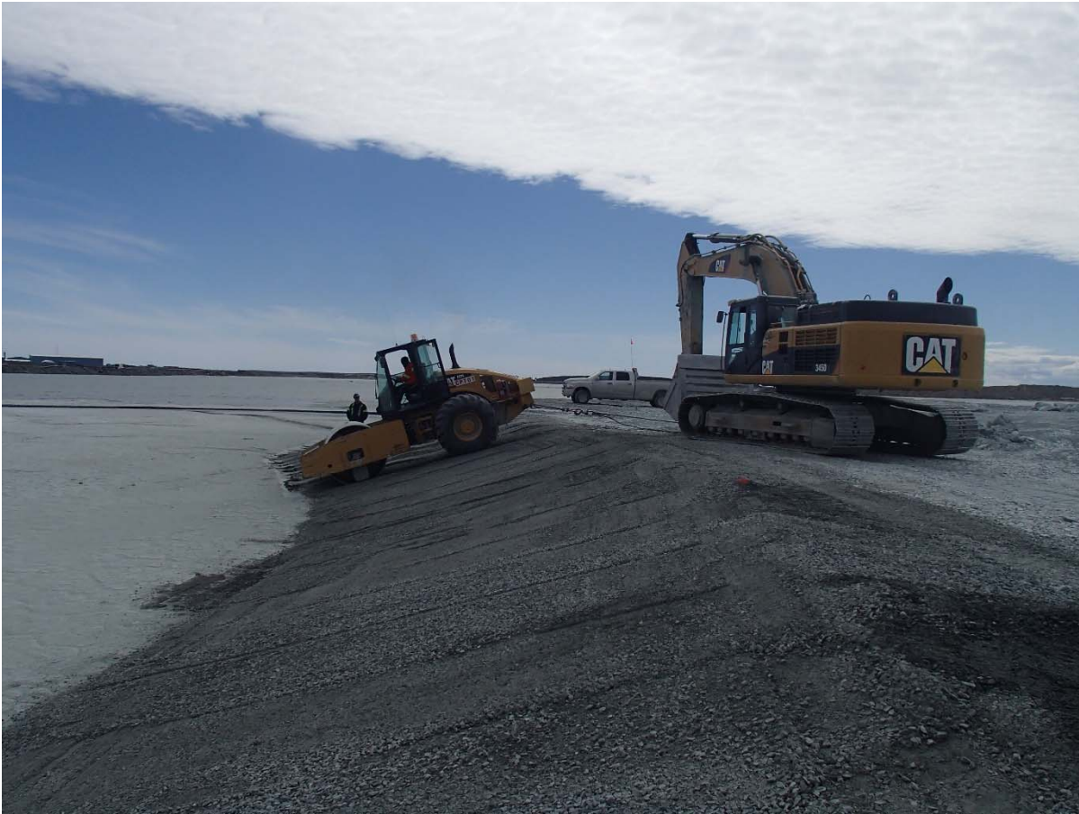
Photograph NCIS-070: From Sta. 1+160/-89 m (approx.), looking S. Compaction of the 0.5 m lift of fine filter between El. 150 and 152 m with a 10-tonne smooth-drum compactor with vibration (4 passes) in the upstream slope from Sta. 1+335 m to 1+100 m.
