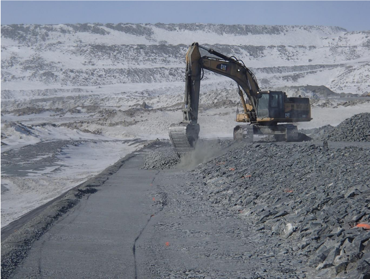
Photograph CD-1832: From Sta 0+280/-25 m, looking N. Placement of a second 0.5 m thick lift of coarse filter from El. 143.5 m to 144 m with an excavator from Sta. 0+175 m to 0+280 m.
