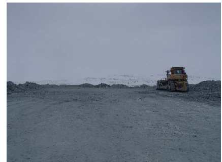
NCIS-009 (2018-05-21). Placement a 2 m thick (approx.) lift of UM rockfill from El. 150 m to El. 152 m (approx.) with a dozer from Sta. 1+880 m to 1+825 m (o.s. unavailable).
