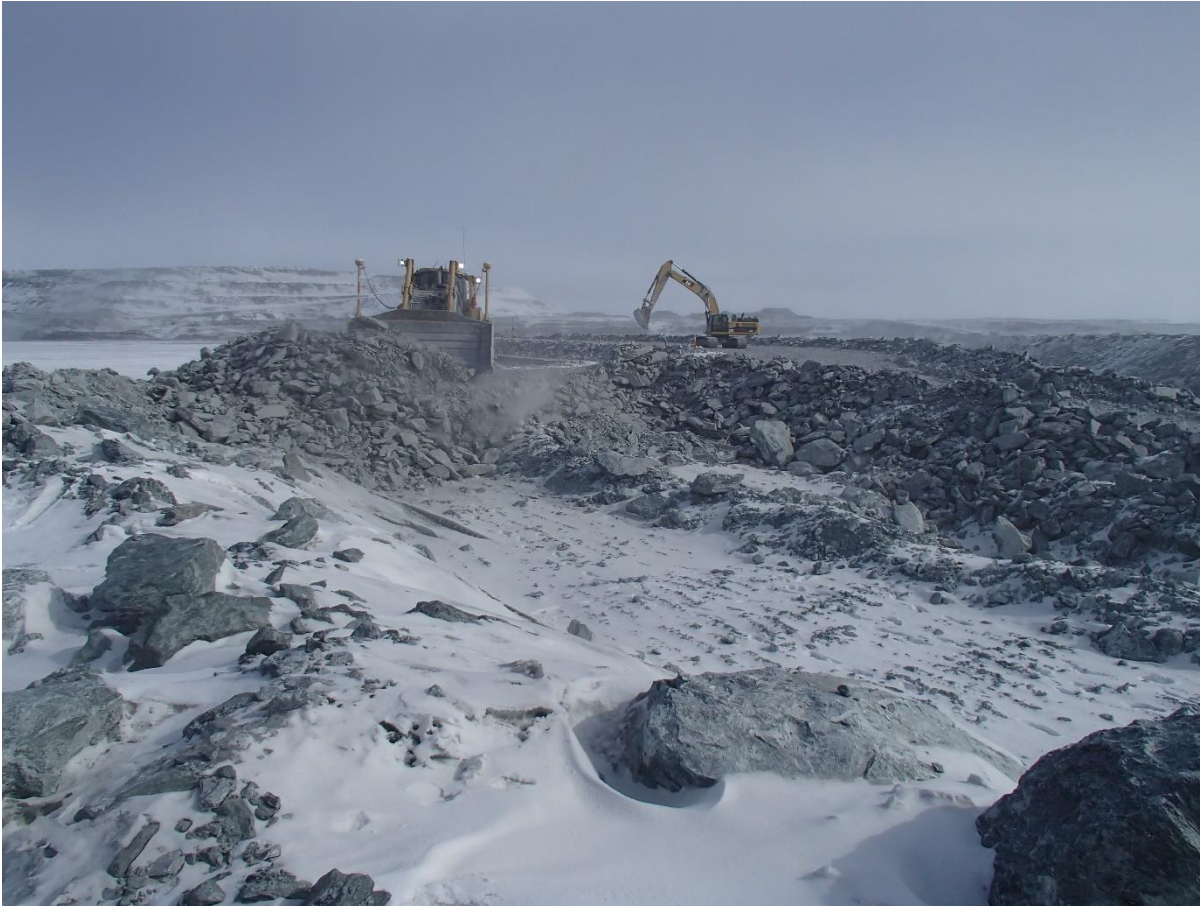
Photograph CD-1822: From Sta. 40+725/+7, looking N. Placement of two 2 m thick (approx.) lifts of intermediate volcanic (IV) rockfill from El. 141 m to El. 145 m from approx. Sta. 40+720 m to 40+750 m (o.s. -10 to +10 m) and profiling of the upstream slope (2H:1V) from El. 143 to 145 m with an excavator between Sta. 0+830 m and 0+980 m.
