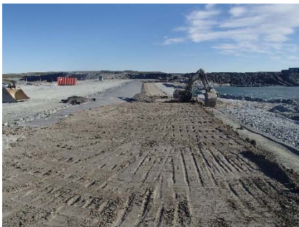
SD3-335 (2018-07-14), looking N from Sta. 20+815/-27 m. Placement of a third 0.5 m thick lift of compacted sieved till on the upstream slope of the upstream toe liner tie-in with an excavator from Sta. 20+760 m to 20+810 m.
