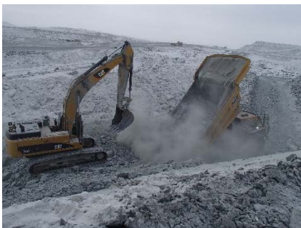
CD-1811 (2018-04-30), looking SE from Sta. 0+985/-11 m. Placement the second, third, fourth and fifth 1 m thick (approx.) lifts of intermediate volcanic (IV) rockfill from approx. Sta. 0+985 to 40+780 m (o.s. -8 to 8 m) with the excavator.
