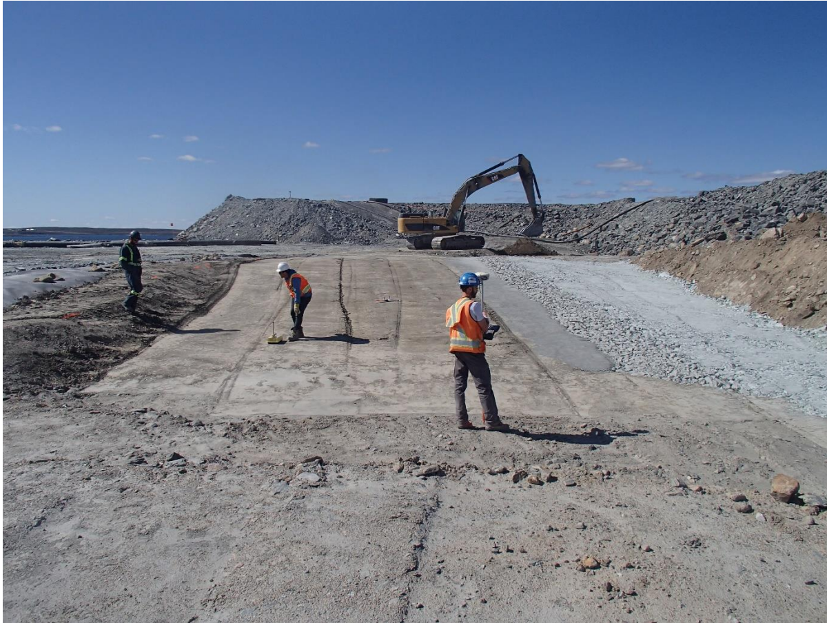
Photograph SD3-342: From Sta. 20+600/-57 m, looking W. View of the compaction test and view of the filling of the depression between SD2 and SD3 with low quality till up to El. 145 m.
