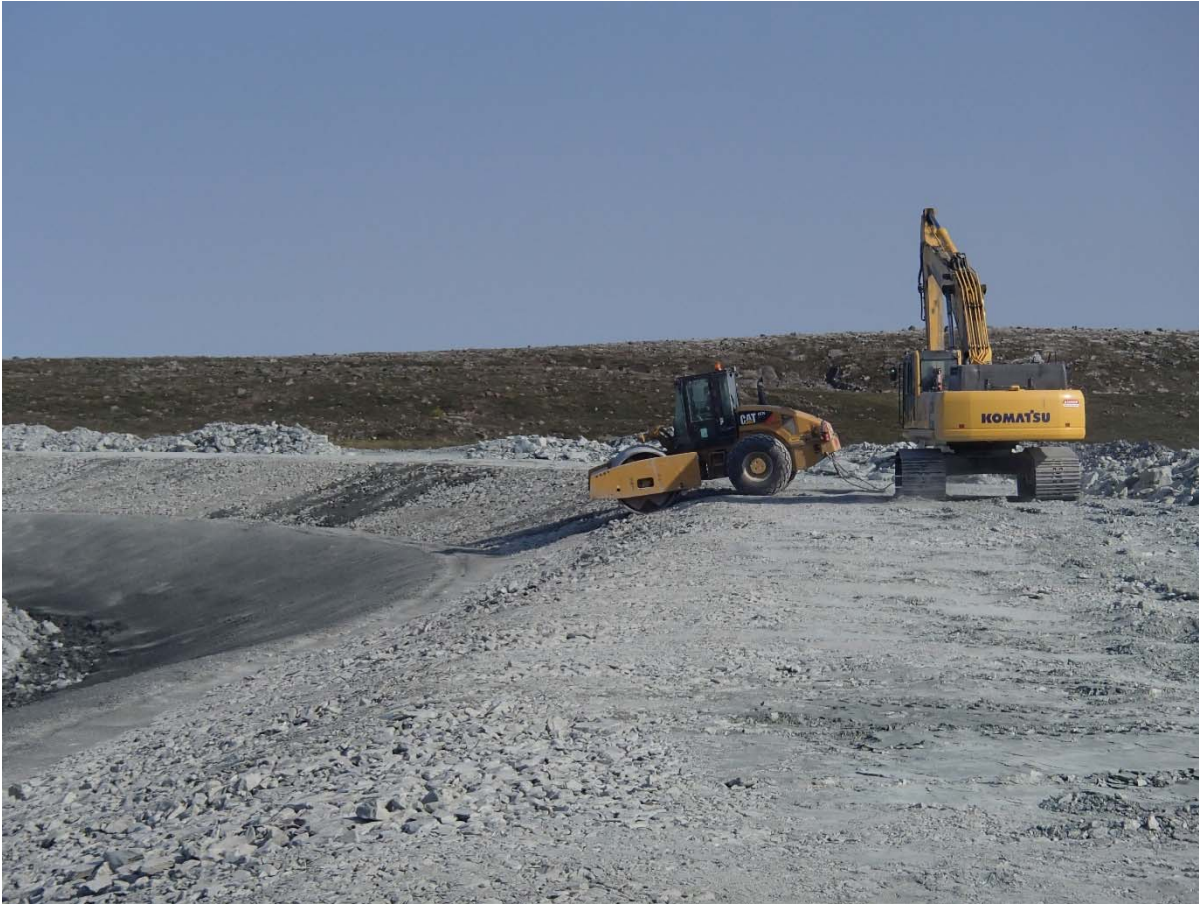
Photograph NCIS-110: From Sta. 2+320/-22 m (approx.), looking N. Compaction of the 0.5 m lift (approx.) of coarse filter between El. 152 m and 154 m with a 10-tonne smooth-drum compactor with vibration (4 passes) in the upstream slope from Sta. 2+293 m to 2+080 m.
