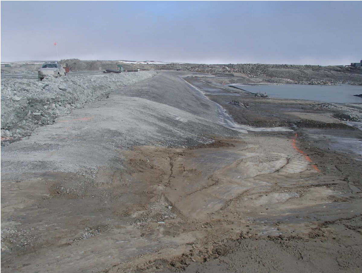
Photograph SD3-307: From Sta. 20+800/-25 m, looking N. View of the liner bedding ready for geosynthetics installation.
