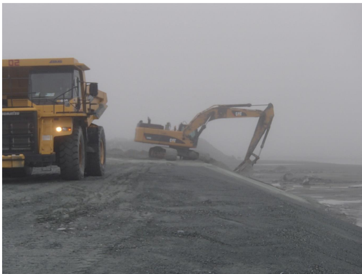
Photograph NCIS-082: From Sta 3+060/-33 m (approx.), looking S. Placement of a 0.5 m thick lift of fine filter over the coarse filter in the upstream slope from El. 150 m to 152 m with an excavator from Sta. 3+120 m to 3+160 m.
