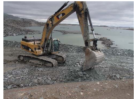
SD3-320 (2018-07-08), looking E from Sta. 20+620/-67 m. Placement of a 1 m thick (approx.) lift of fine IV rockfill over the compacted till in the upstream slope from El. 142 m to 144 m with an excavator from Sta. 20+600 m to 20+610 m.
