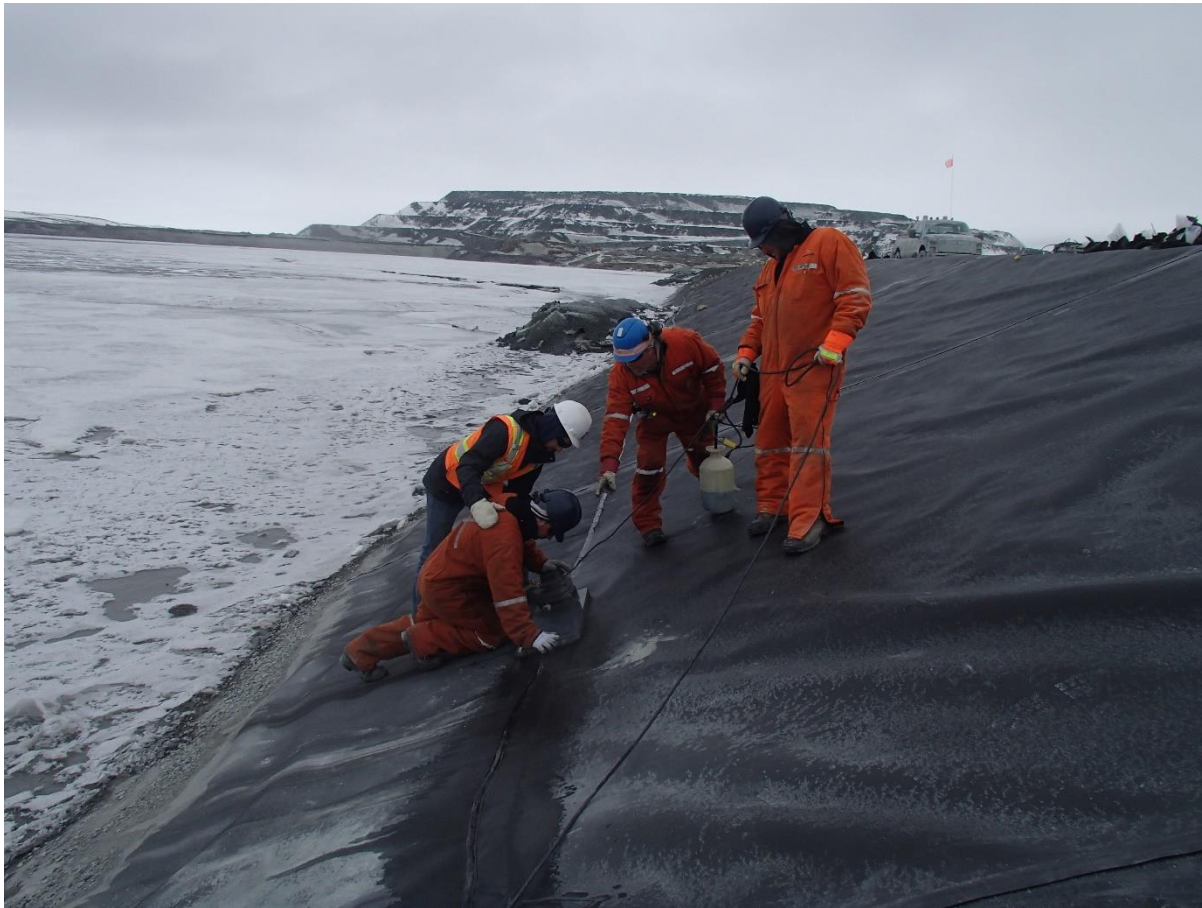
Photograph CD-1875: From Sta. 0+835/-26 m, looking N. View of a vacuum box testing.
