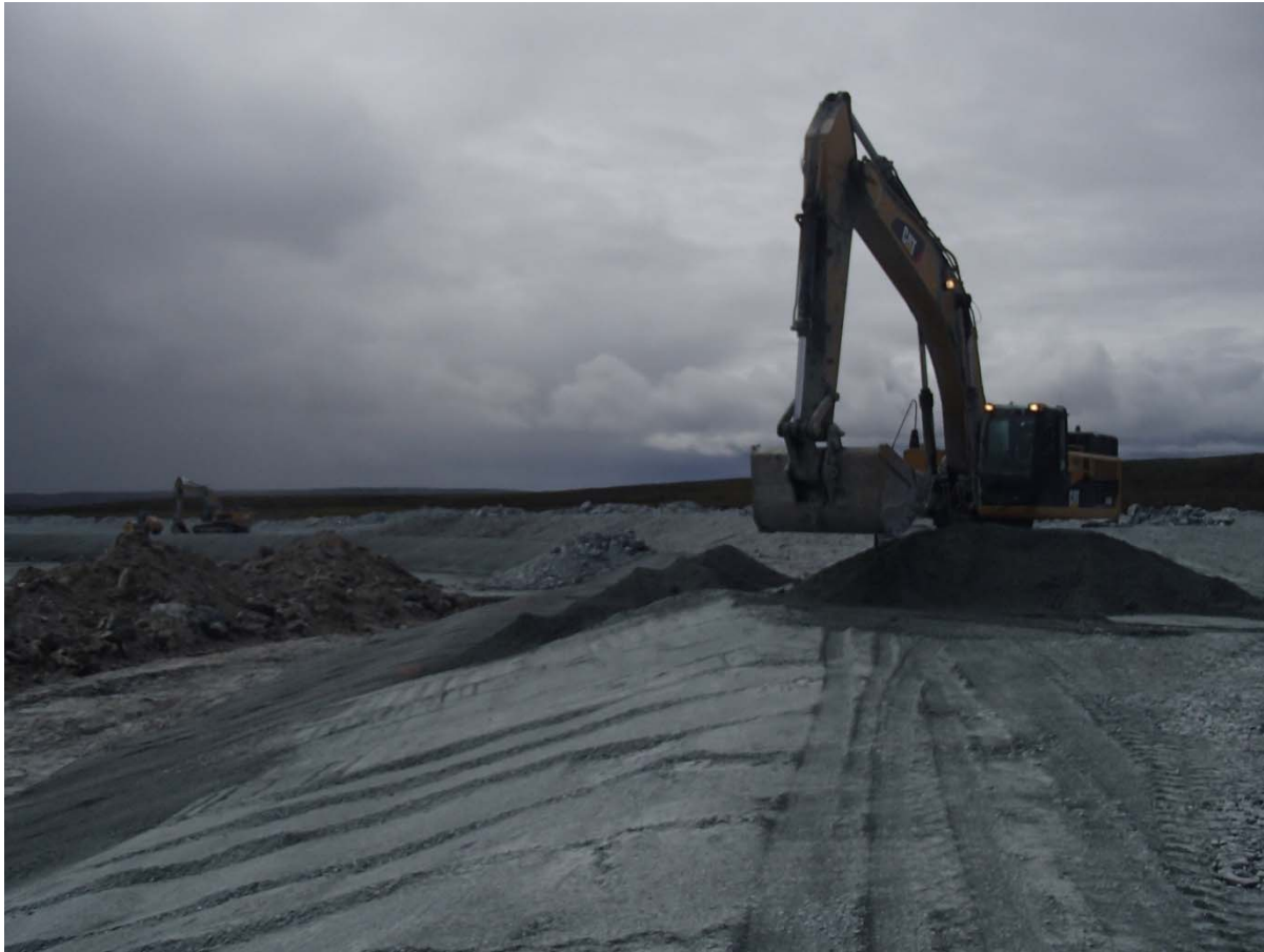
Photograph NCIS-135: From Sta. 1+860/-12 m (approx.), looking SW. Placement of a 0.5 m thick lift of fine filter in the upstream slope from El. 152 m to 154 m with an excavator from Sta. 1+830 m to 1+700 m.
