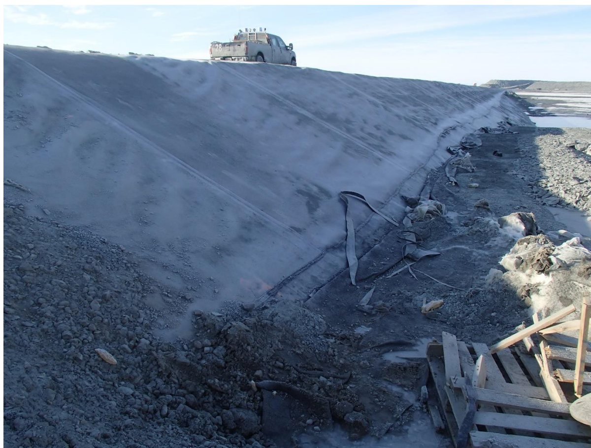
Photograph CD-1892: From Sta. 0+155/-32 m, looking S. View of the liner panel 933 overlapping the underlying liner that has been cut at around Sta. 0+160 m to drain the water.
