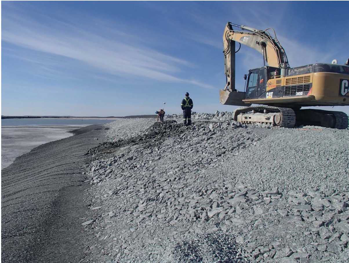
Photograph NCIS-097: From Sta. 1+180/-75 m (approx.), looking SW. Placement of a 0.5 m thick lift of coarse filter in the upstream slope from El. 150 m to 152 m with an excavator from Sta. 1+200 m to 1+113 m.
