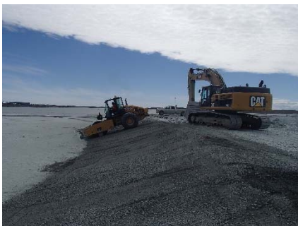
NCIS-070 (2018-07-01), looking S from Sta. 1+160/-89 m. Compaction of the 0.5 m lift of fine filter between El. 150 and 152 m with a 10-tonne smooth-drum compactor with vibration (4 passes) in the upstream slope from Sta. 1+335 m to 1+100 m.
