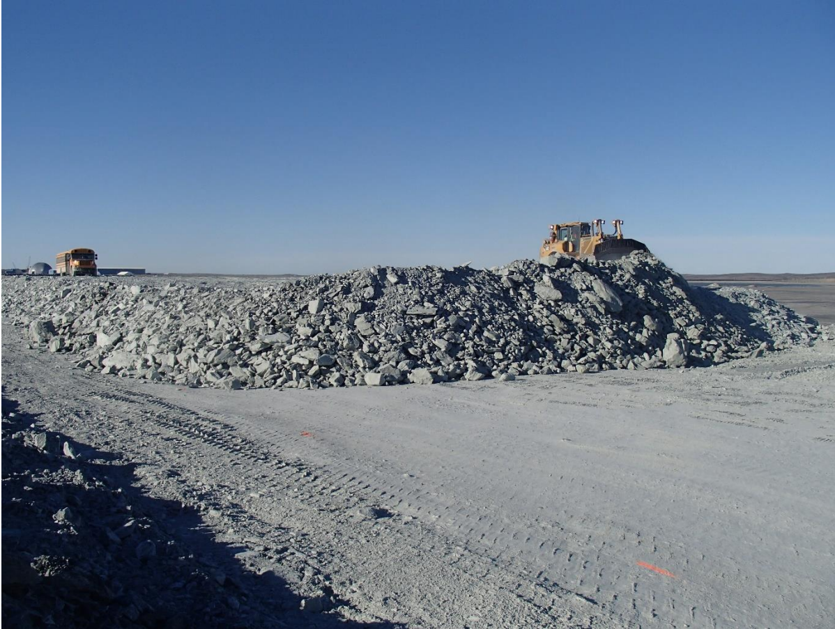
Photograph NCIS-091: From Sta 2+330/+13 m (approx.), looking S. Placement of a 2 m thick (approx.) lift of UM rockfill from El. 152 m to El. 154 m (approx.) with a dozer from Sta. 2+370 m to 2+290 m (+9 m to -22 m). The material is of good quality and is well graded.
