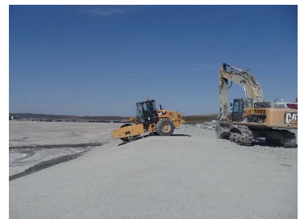
NCIS-126 (2018-07-27), looking W from Sta. 1+140/-98 m (approx.). Compaction of the 0.5 m lift (approx.) of fine filter between El. 150 m and 152 m with a 10-tonne smooth-drum compactor with vibration (4 passes) in the upstream slope from Sta. 1+240 m to 1+100 m.
