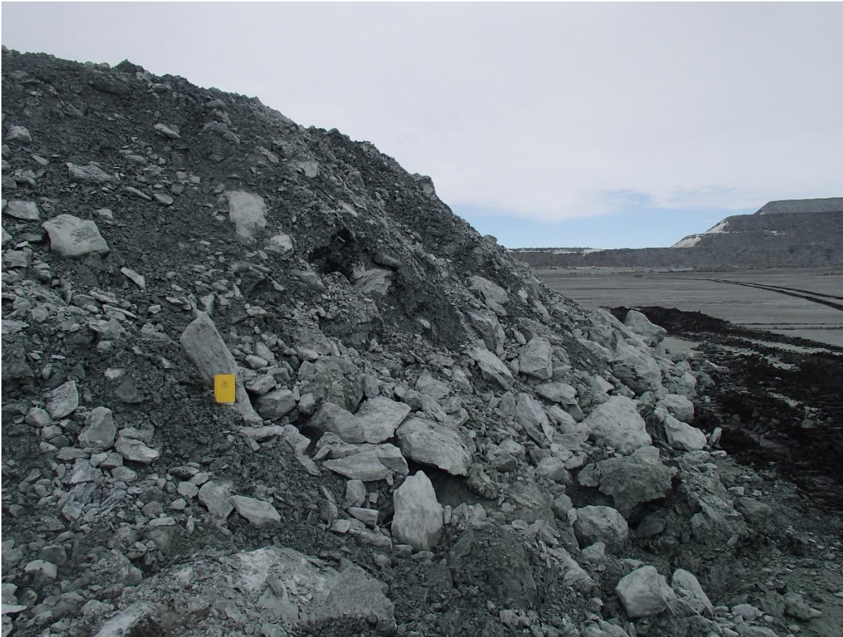
Photograph NCIS-028: From Sta. 1+340/+3 m, looking E. View of the UM rockfill lift approximately 3.2 m thick.
