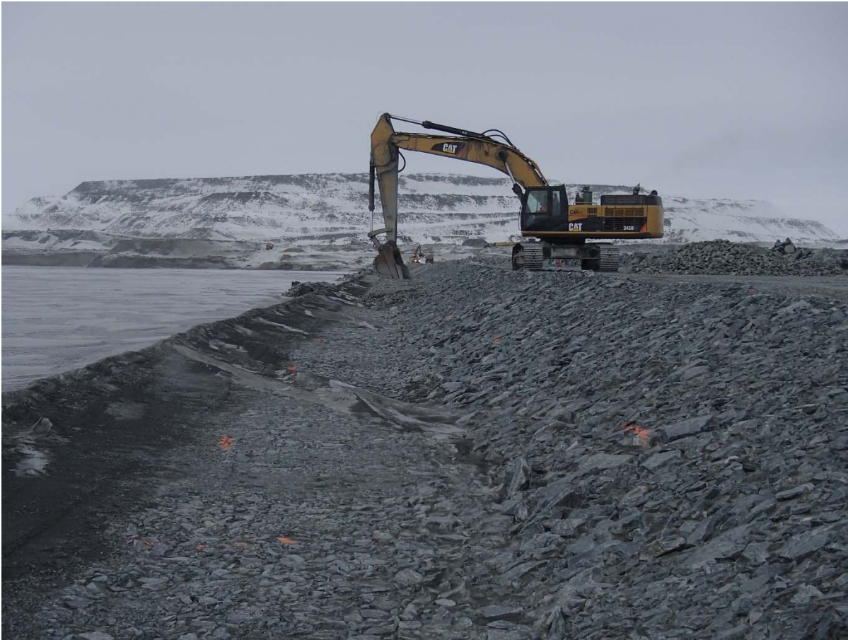
Photograph CD-1837: From Sta. 0+940/-25 m, looking N. Placement of a second 0.5 m thick lift of coarse filter from El. 143.5 m to 144 m with an excavator from Sta. 0+290 to 0+500 m and from Sta. 0+835 to 0+930 m.
