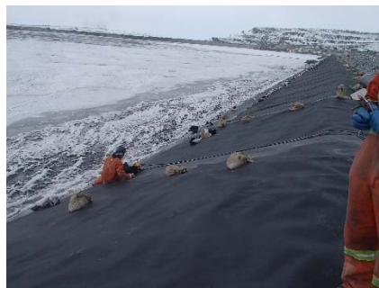
CD-1866 (2018-05-25), looking NW from Sta. 0+940/-25 m. Installation of the LLDPE liner on the upstream slope 2H:1V between El. 143 m and 145 m from Sta. 0+950 m to 0+935 m (panel numbers 818 and 819).
