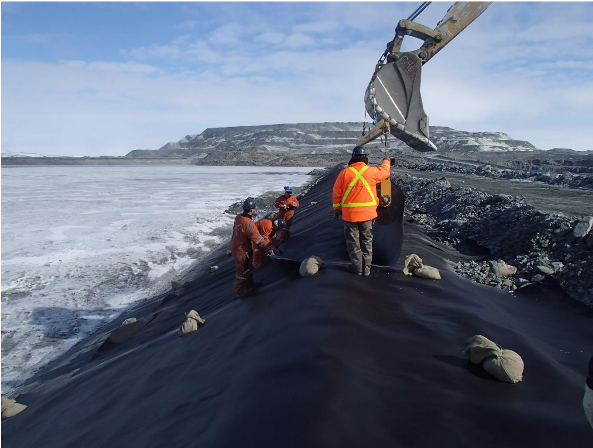
Photograph CD-1878: From Sta. 0+720/-24 m, looking N. Installation of the LLDPE liner on the upstream slope 2H:1V between El. 143 m and 145 m from Sta. 0+740 m to 0+610 m (panel numbers 849 to 867).
