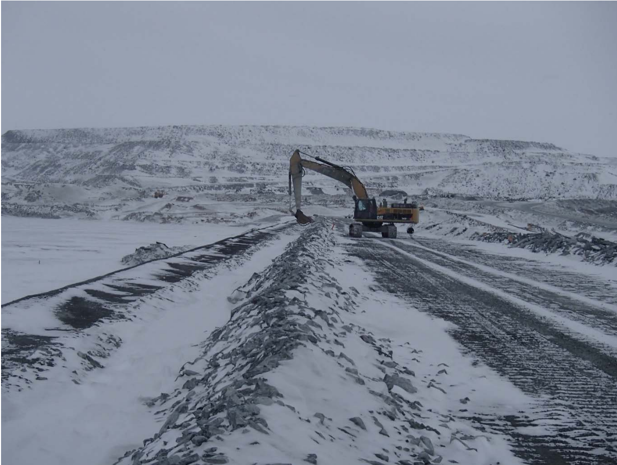
Photograph CD-1857: From Sta. 0+700/-20 m, looking N. Snow removal in the anchoring trench with an excavator between Sta. 0+170 m and 40+780 m.
