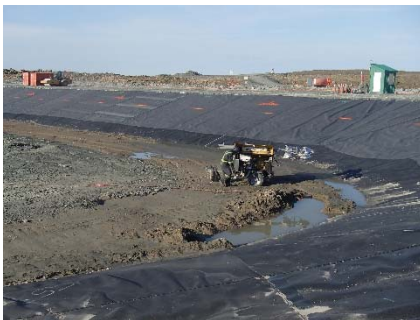
SD3-321 (2018-07-09), looking SW from Sta. 20+610/-56 m. Water ponding at El. 142m on the compacted sieved till layer of the upstream toe liner tie-in at approx. Sta. 20+620 m to 20+630 m was pumped.
