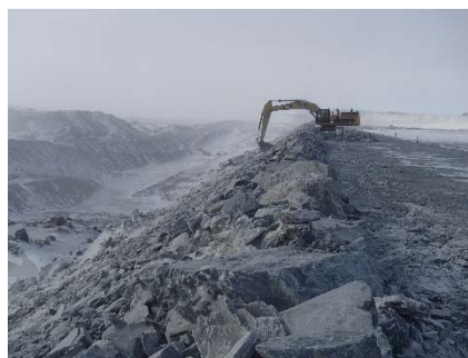
CD-1821 (2018-05-04), looking S from Sta. 0+175/+3 m. Profiling of the downstream slope (1.5H:1V) from El. 143 to 145 m with an excavator between Sta. 0+250 m and 0+330 m.
