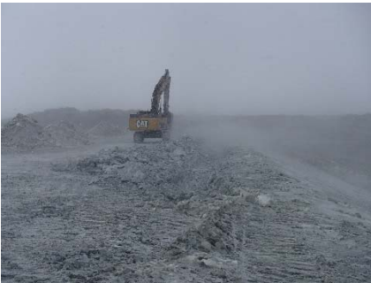
SD3-300 (2018-05-16), looking NW from Sta. 20+790/-33 m. Excavation of the LLDPE geomembrane crest anchoring trench with an excavator from Sta. 20+675 m to 20+780 m.
