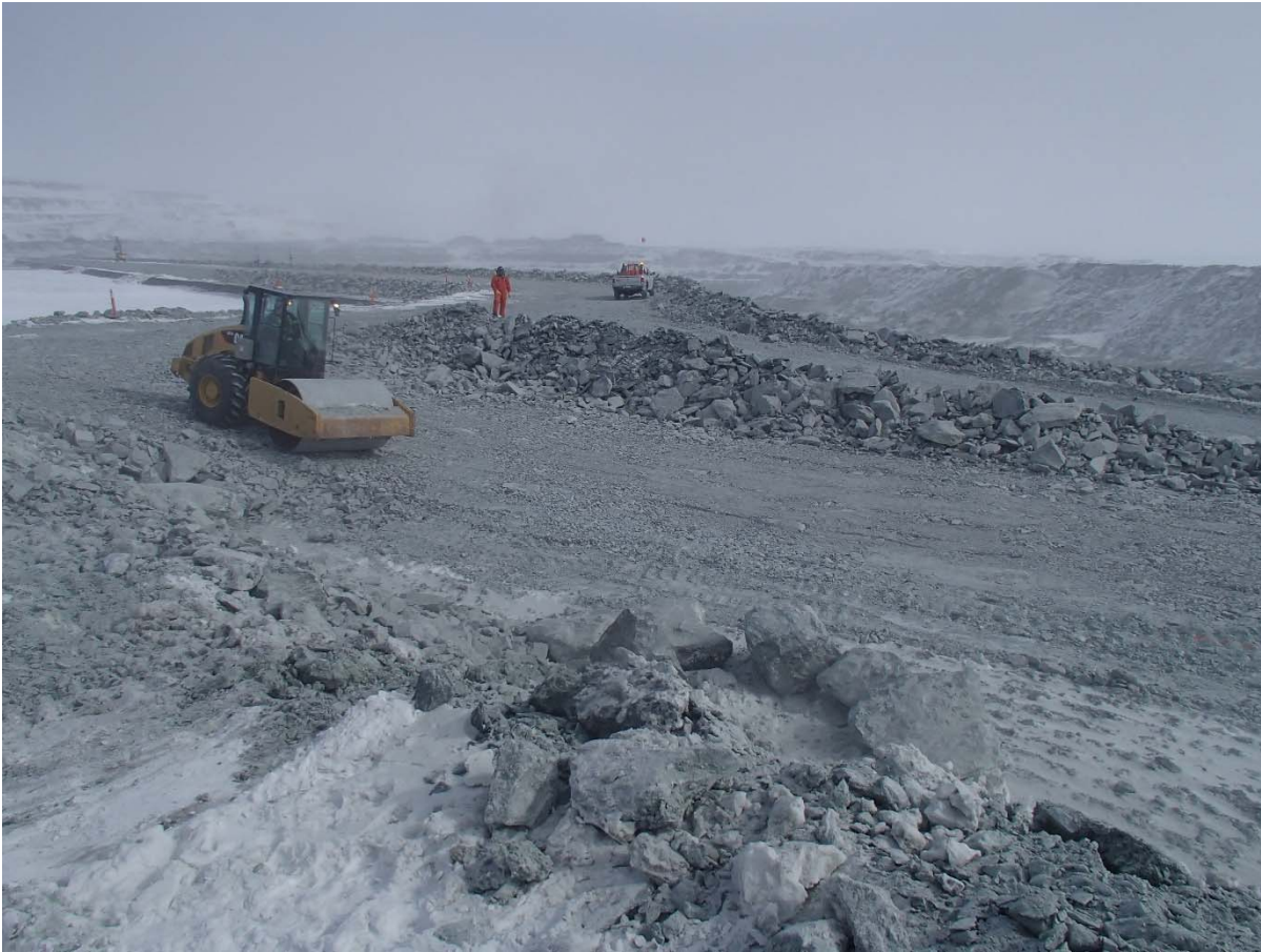
Photograph CD-1823: From Sta. 0+175/+8, looking NE. Compaction of the two 2 m lifts (approx.) of intermediate volcanic (IV) rockfill at El. 143 and at El. 145 m with a 10-tonne smooth-drum compactor with vibration (6 passes) from Sta. 40+720 m to 40+750 m (o.s. -10 to +10 m).
