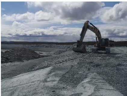
NCIS-133 (2018-07-29), looking W from Sta. 1+820/-28 m (approx.). Placement of a 0.5 m thick lift of coarse filter in the upstream slope from El. 152 m to 154 m with an excavator from Sta. 1+890 m to 1+826 m.
