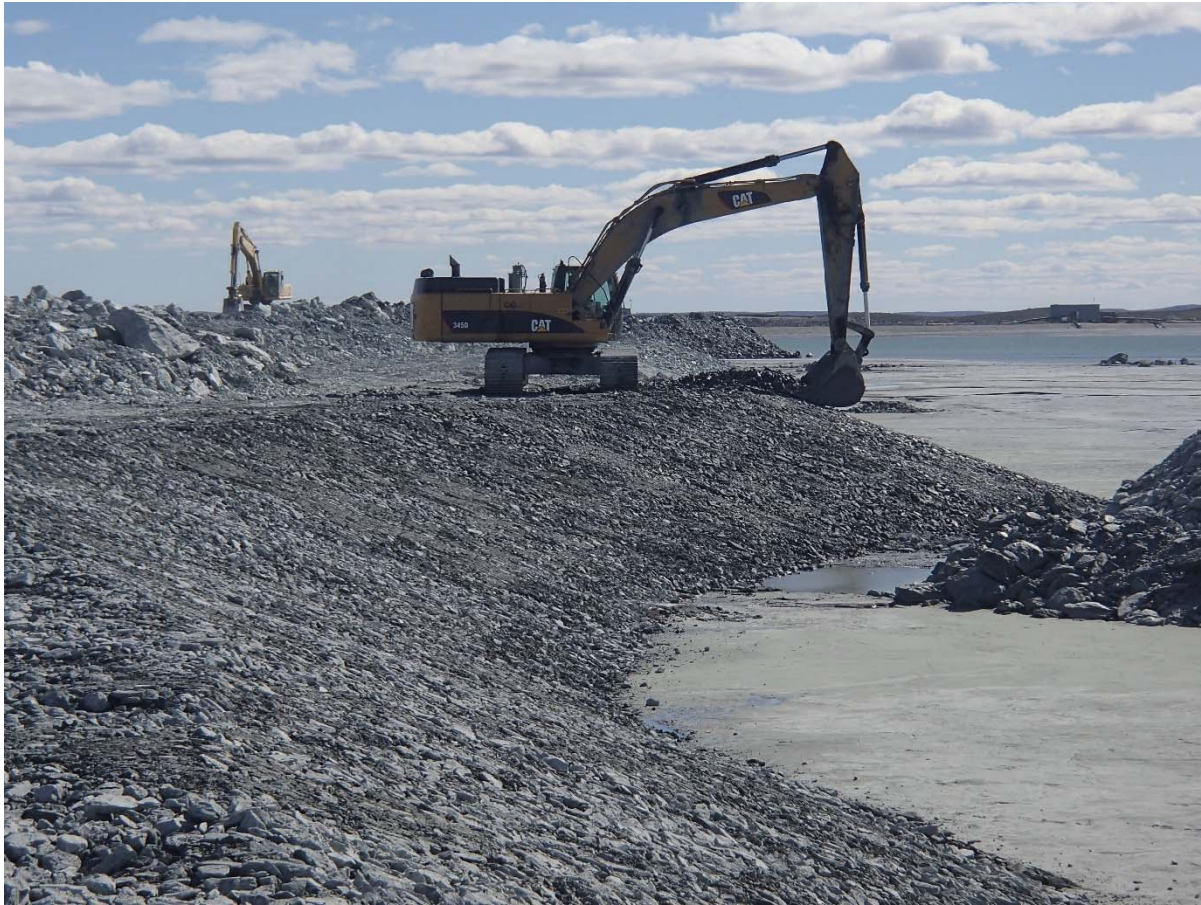
Photograph NCIS-075: From Sta. 2+860/-36 m (approx.), looking S. Placement of a 0.5 m thick lift of coarse filter in the upstream slope from El. 150 m to 152 m with an excavator from Sta. 2+815 m to 2+980 m.
