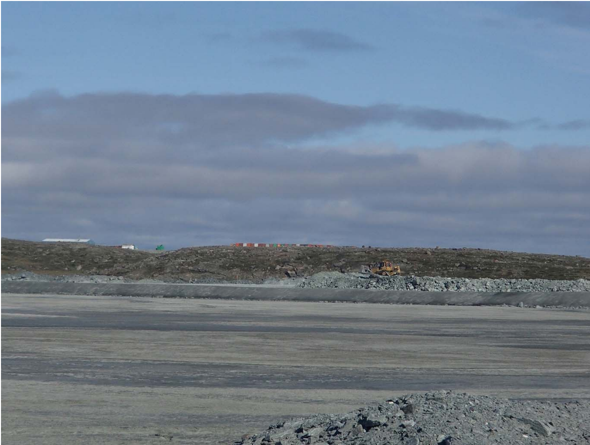
Photograph NCIS-106: From Sta. 2+620/-35 m (approx.), looking NW. Placement of a 2 m thick (approx.) lift of UM rockfill from El. 152 m to El. 154 m (approx.) with a dozer from Sta. 1+947 m to 1+863 m (+14 m to -26 m). The material is of good quality and is well graded.
