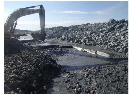
NCIS-123 (2018-07-27), looking S from Sta. 3+340/+33 m (approx.). Excavation of a 1 m (approx.) deep sump (south sump) in the tailings with an excavator from Sta. 3+345 m to 3+365 m (o.s. +24 to +32 m).
