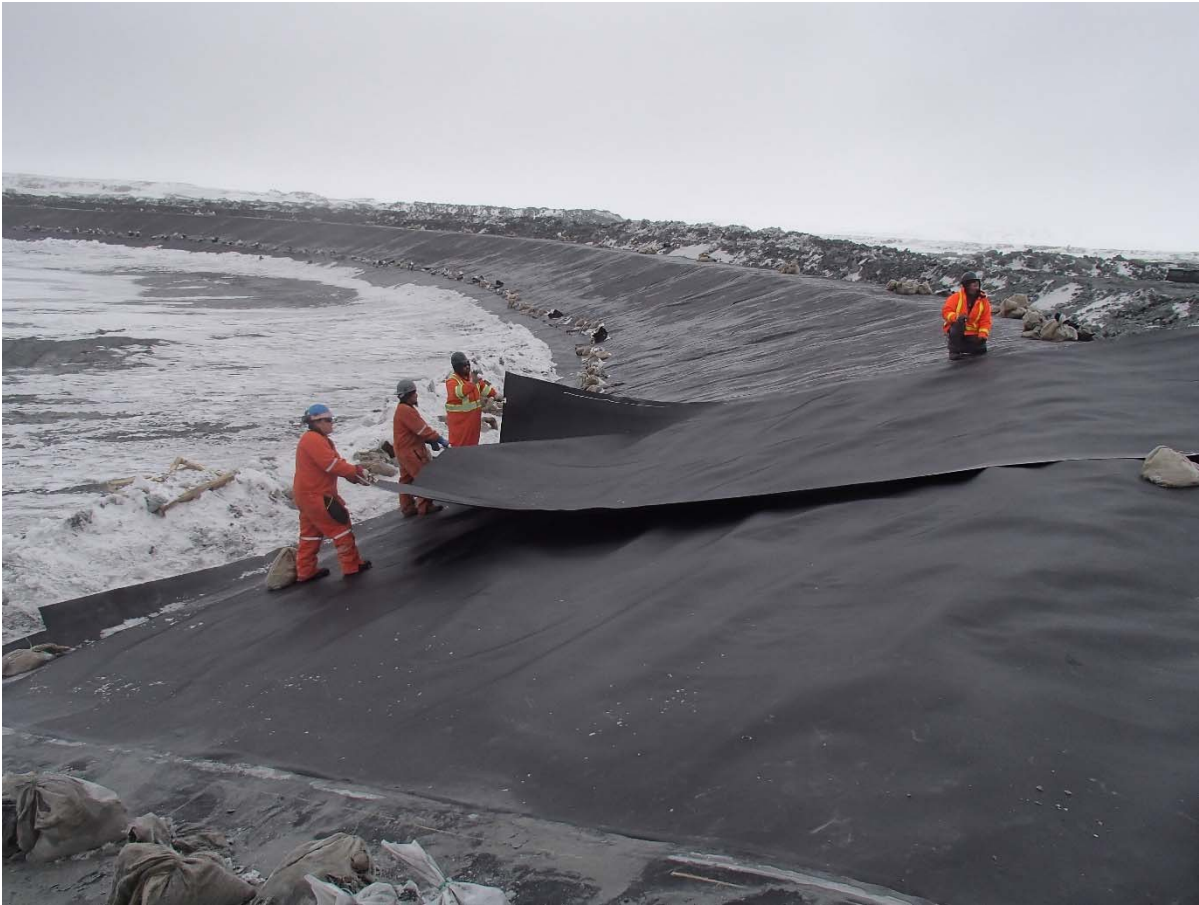
Photograph CD-1861: From Sta. 40+680/-28 m, looking NE. Installation of the LLDPE liner on the upstream slope 3H:1V (SD5 side) to 2H:1V (Central Dike side) between El. 143 m and 145 m from Sta. 40+680 m to 0+950 m (panel numbers 802 to 817).
