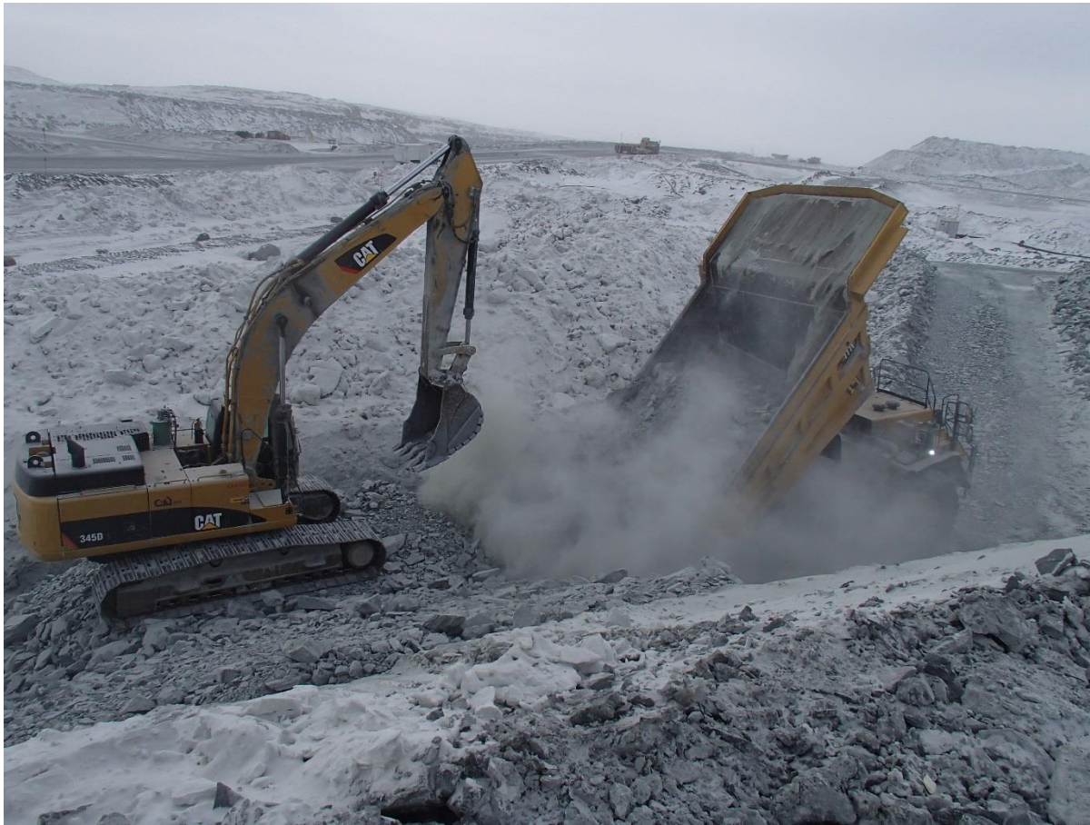
Photograph CD-1811: From Sta. 0+985/-11 m looking SE. Placement the second, third, fourth and fifth 1 m thick (approx.) lifts of intermediate volcanic (IV) rockfill from approx. Sta. 0+985 to 40+780 m (o.s. -8 to 8 m) with the excavator.
