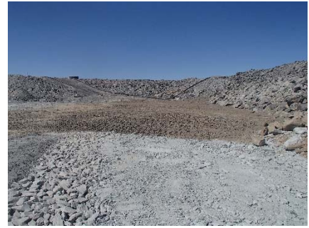
SD3-343 (2018-07-16), looking W from Sta. 20+590/-40 m. View of the depression between SD2 and SD3 backfilled with low quality till up to El. 145 m.
