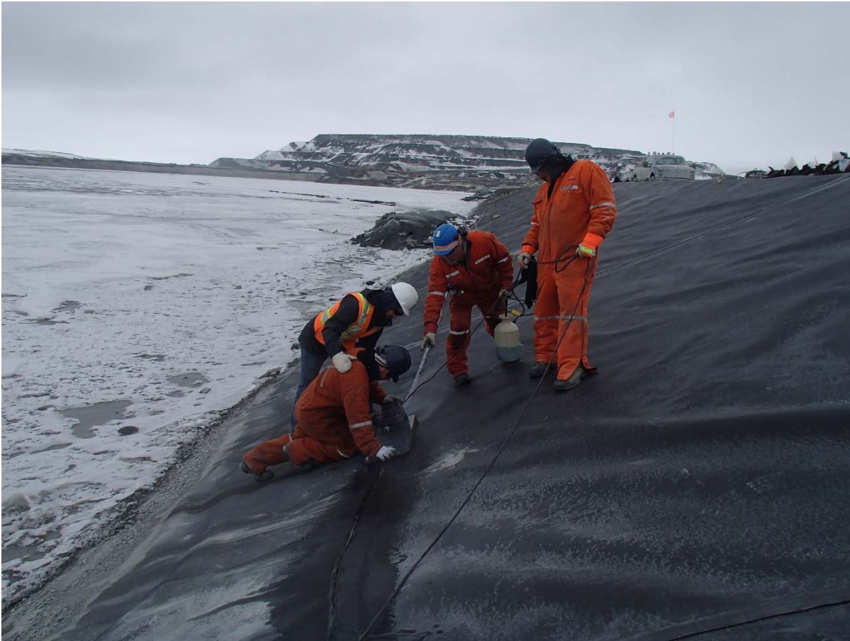
Photograph CD-1875: From Sta. 0+835/-26 m, looking N. View of a vacuum box testing.
