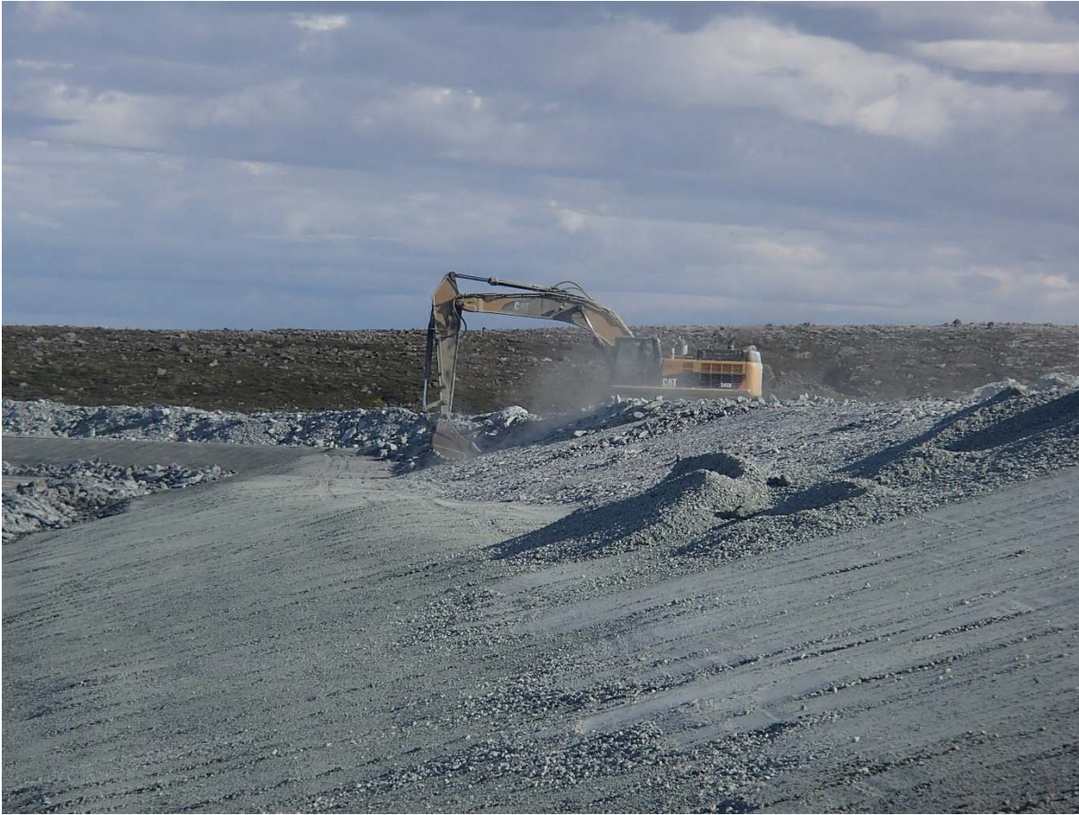
Photograph NCIS-108: From Sta. 2+490/-32 m (approx.), looking N. Profiling of the upstream slope (3H:1V) from El. 152 to 154 m with an excavator from Sta. 2+159 m to 2+409 m.
