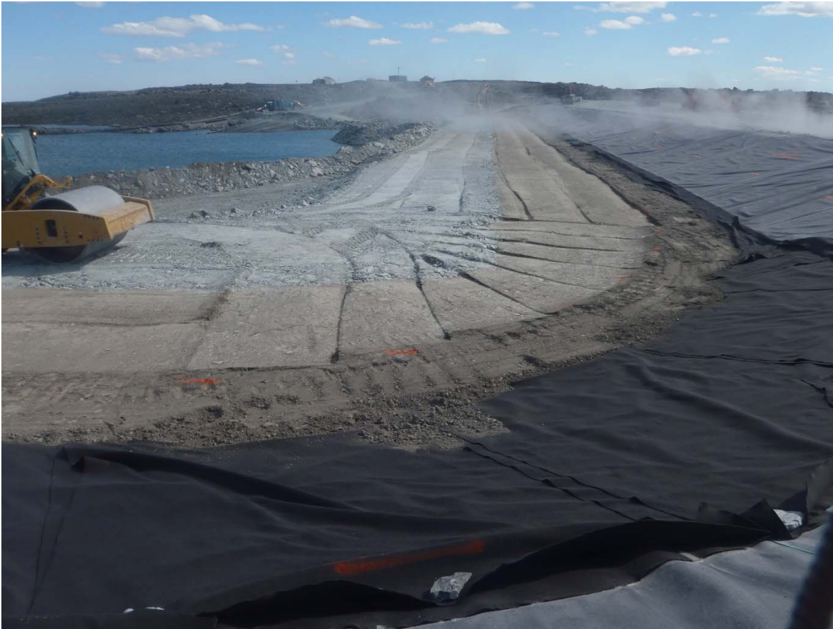
Photograph SD3-331: From Sta. 20+610/-43 m, looking S. Compaction of the 0.5 m lift of low quality till (0-150 mm) at El. 143 m with a 10-tonne smooth-drum compactor with vibration (4 passes) from Sta. 20+610 m to 20+760 m.
