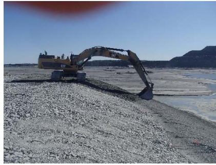
NCIS-101 (2018-07-20), looking N from Sta. 1+120/-89 m (approx.). Placement of a 0.5 m thick lift of fine filter in the upstream slope from El. 150 m to 152 m with an excavator from Sta. 1+113 m to 1+205 m.
