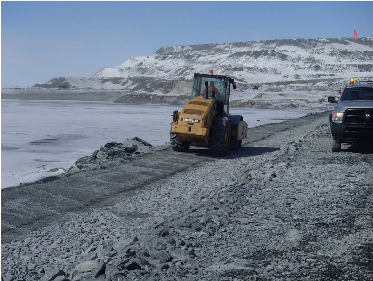
Photograph CD-1840: From Sta. 0+575/-15 m, looking NW. Compaction of the second 0.5 m lift (approx.) of fine and coarse filters material at El. 144 m with a 10-tonne smooth-drum compactor with vibration (4 passes) from Sta. 0+500 m to 40+730 m.
