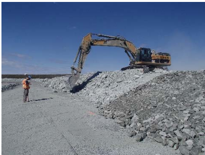
NCIS-103 (2018-07-20), looking NE from Sta. 2+420/-27 m (approx.). Profiling of the upstream slope (3H:1V) from El. 152 to 154 m with an excavator from Sta. 2+400 m to 2+410 m. Oversize boulders were removed.
