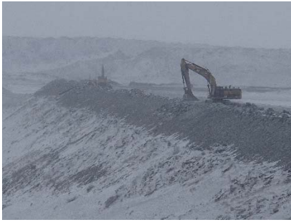
CD-1850 (2018-05-13), looking SW from Sta. 0+160/+20 m. Profiling of the downstream slope (1.5H:1V) from El. 143 to 145 m with an excavator between Sta. 0+440 m and 0+530 m and between Sta. 0+745 m and 0+835 m.
