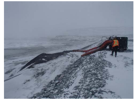
CD-1828 (2018-05-06), looking N from Sta. 0+410/-22 m. Defrosting of the deposition point finger materials with two Frost Fighters at Sta. 0+390 m.
