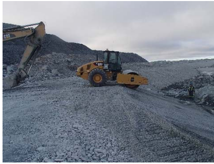
NCIS-074 (2018-07-03), looking SE from Sta. 2+750/-37 m. Compaction of the 0.5 m lift (approx.) of fine filter between El. 150 and 152 m with a 10-tonne smooth-drum compactor (4 passes) in the upstream slope from Sta. 2+810 m to 2+095 m.
