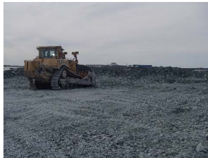
NCIS-041 (2018-06-24), looking S from Sta. 1+220/-7 m. Placement of a 1.5 to 2 m thick (approx.) lift of UM rockfill from El. 148 m to El. 150 m (approx.) with a dozer from Sta. 1+197 m to 1+150 m (-7 m to -41 m).
