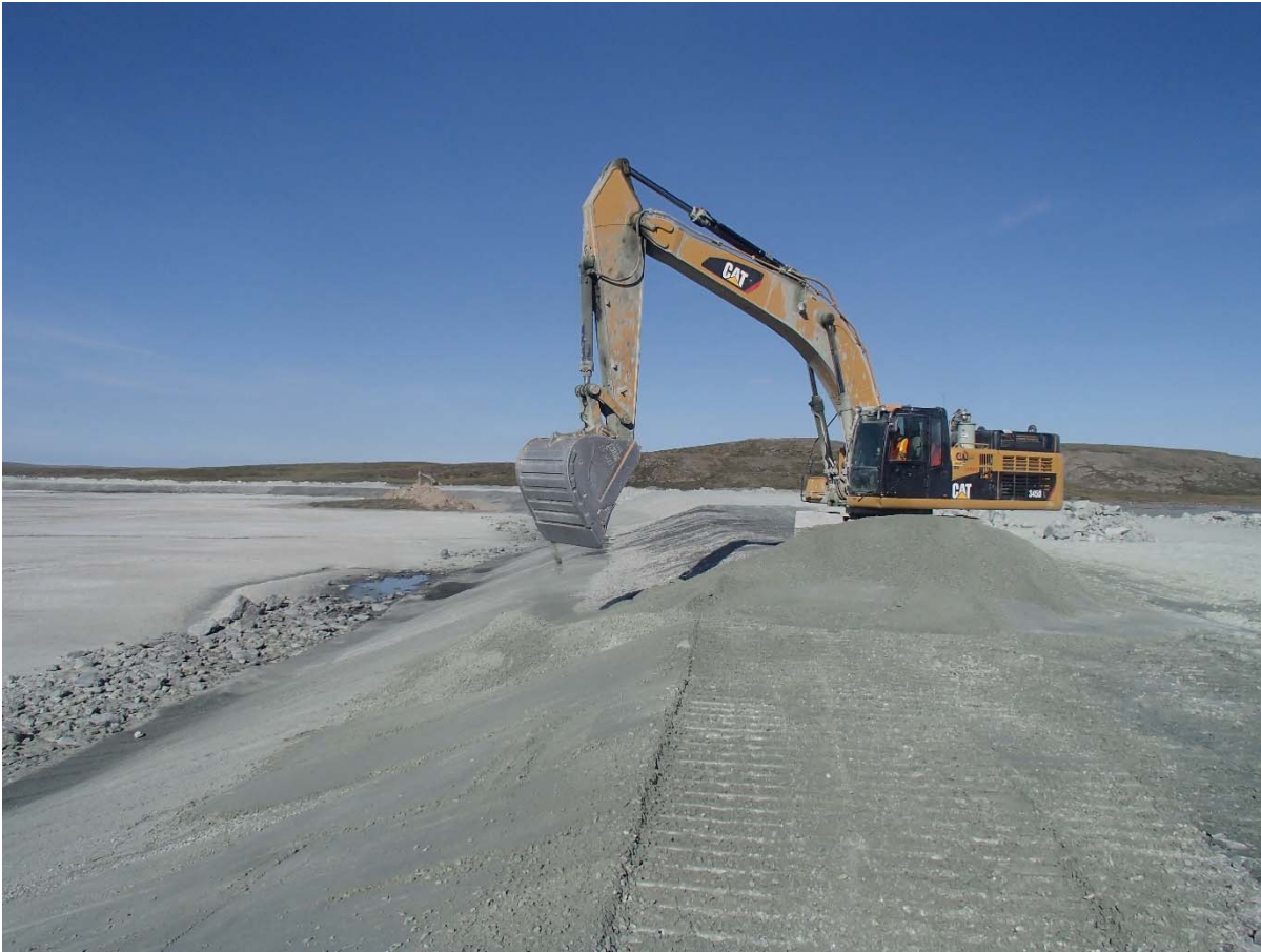
Photograph NCIS-117: From Sta. 2+050/-25 m (approx.), looking SW. Placement of a 0.5 m thick lift of fine filter in the upstream slope from El. 152 m to 154 m with an excavator from Sta. 2+090 m to 1+890 m.
