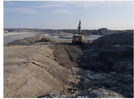
SD3-326 (2018-07-11), looking N from Sta. 20+820/-34 m. Placement of the 0.5 m thick lift of low class till, fine filter, coarse filter and fine rockfill on the upstream slope of the upstream toe liner tie-in with an excavator from Sta. 20+780 to 20+810 m.
