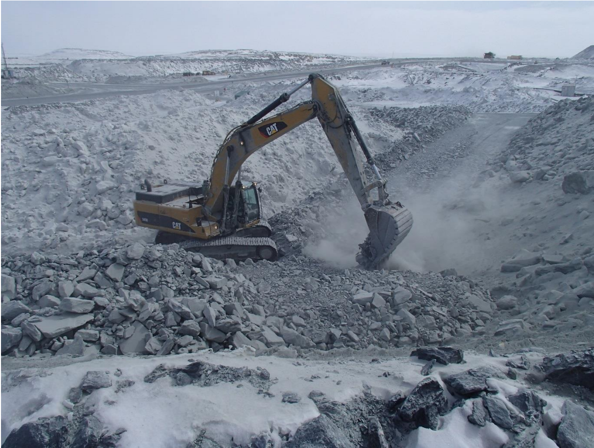
Photograph CD-1812: From Sta. 0+985/-11 m looking SE. Placement of intermediate volcanic (IV) rockfill on the existing downstream slope up to approx. El. 140 m, from approx. Sta. 0+985 to 40+780 m.
