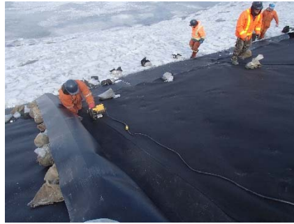
CD-1869 (2018-05-27), looking W from Sta. 0+915/-30 m. Installation of the geotextile on the upstream slope 2H:1V between El. 143 m and 145 m from Sta. 0+935 m to 0+900 m.
