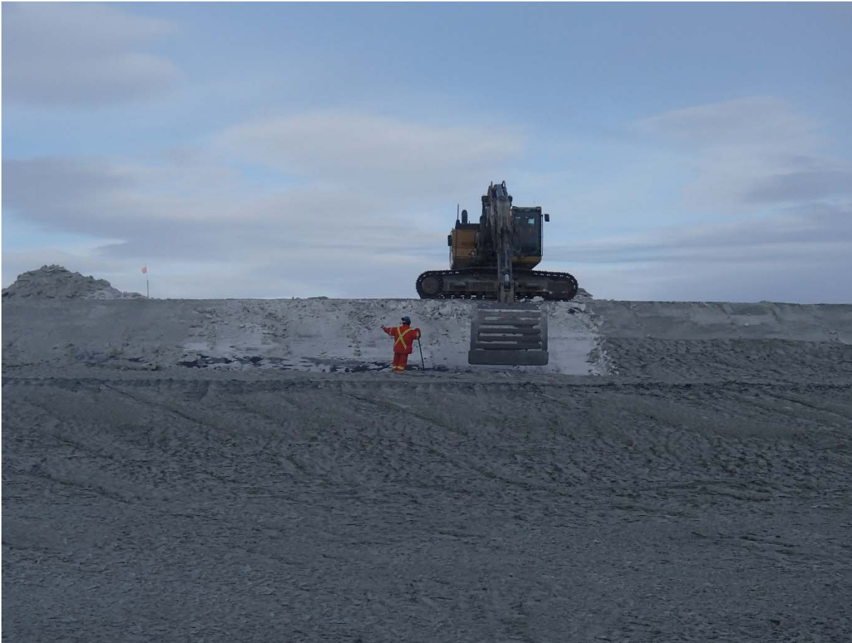
Photograph SD3-298: From Sta. 20+680/-88 m, looking S. Removal of snow on the upstream slope of SD3 above El. 142 m, from Sta. 20+620 m to 20+780 m.
