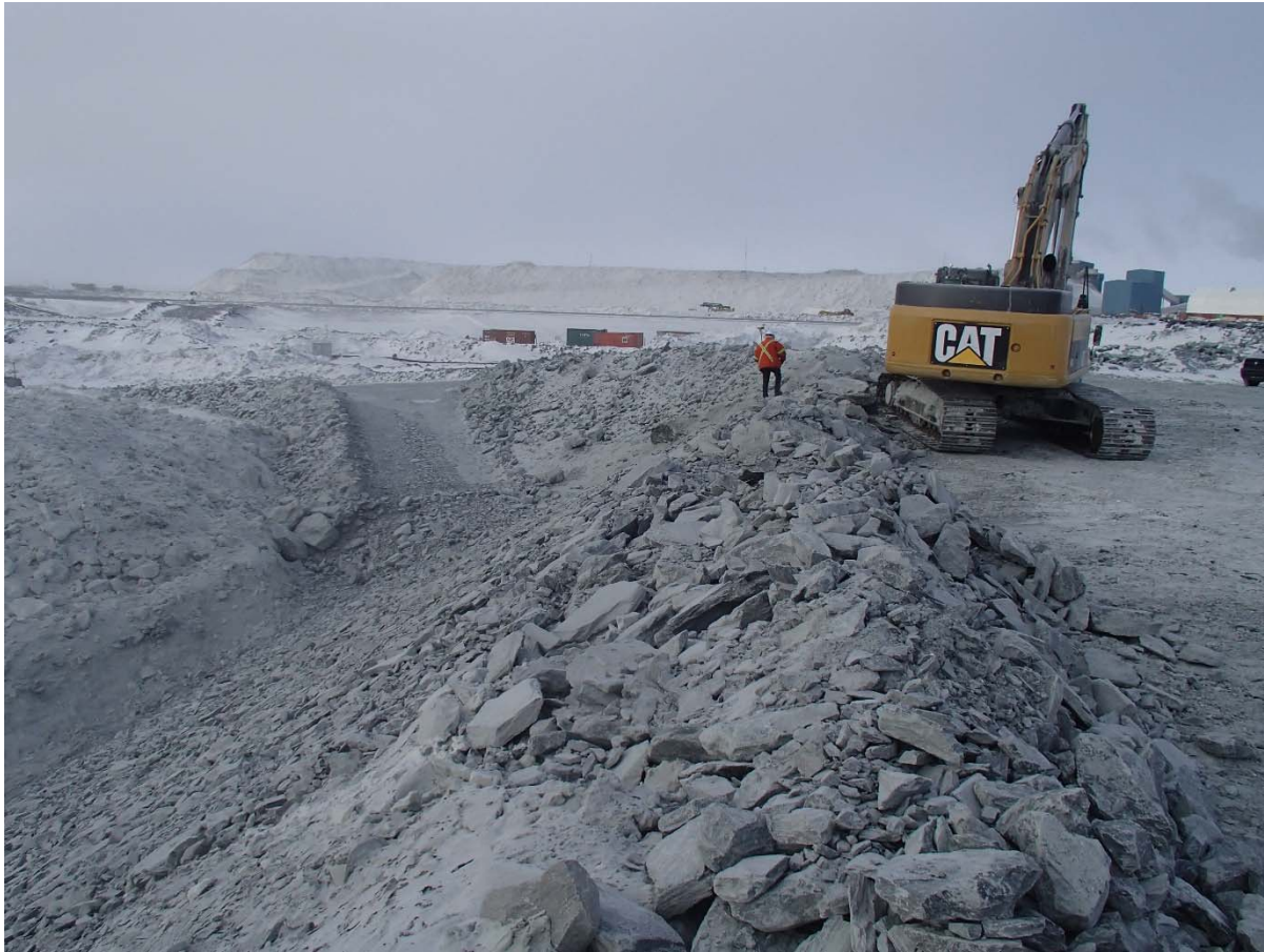
Photograph CD-1813: From Sta. 0+980/-2, looking S. Placement of intermediate volcanic (IV) rockfill on the existing downstream slope up to approx. El. 143 m, from approx. Sta. 0+980 to 40+780 m.
