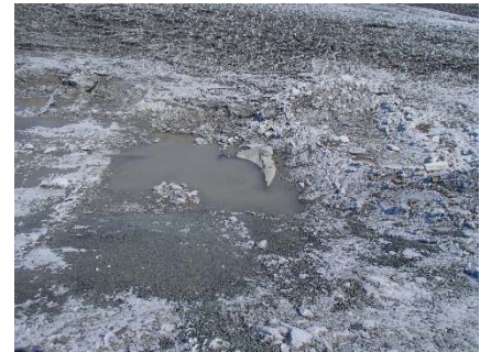
SD3-302 (2018-05-18), looking NE from Sta. 20+595/-42 m. View of water ponding on the first compacted sieved till layer of upstream toe liner tie-in. A portion of exposed damaged LLDPE liner is visible.
