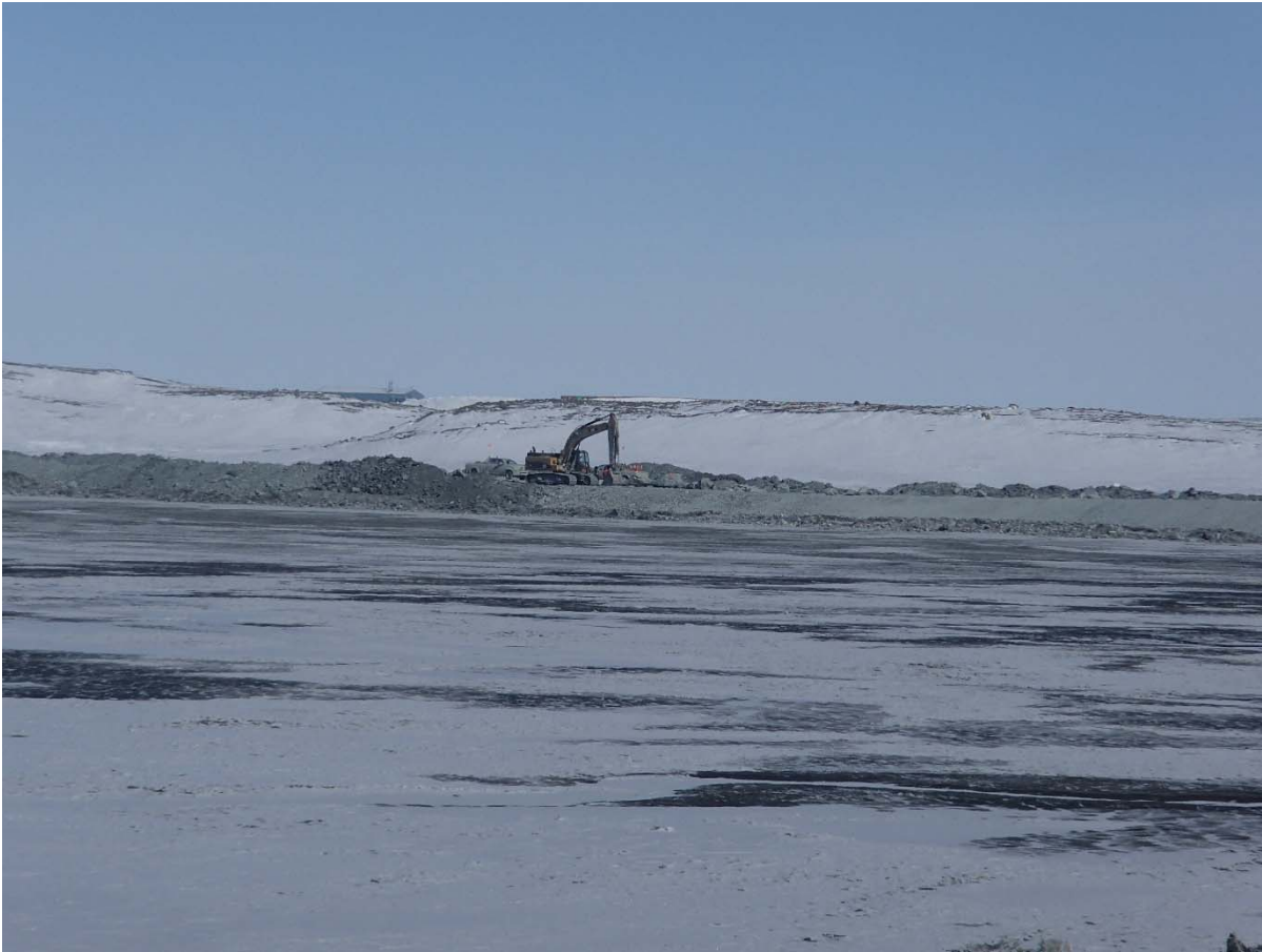
Photograph NCIS-018: From Sta. 2+310 m (approx.), looking NW. Profiling of the upstream slope (3H:1V) from El. 150 to 152 m with an excavator from Sta. 1+989 m to 1+860 m.
