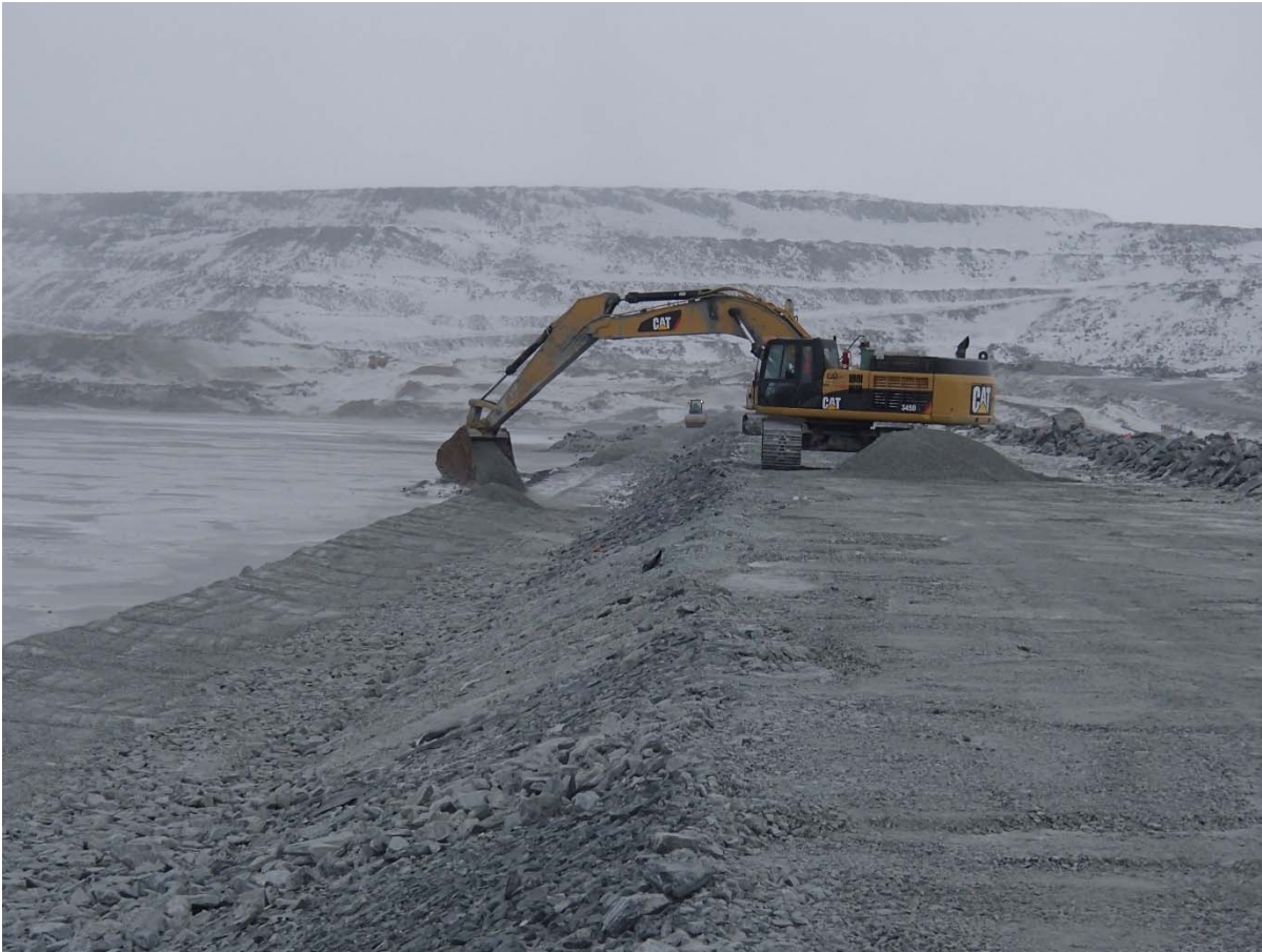
Photograph CD-1836: From Sta. 0+830/-20 m, looking N. Placement of a first 0.5 m thick lift of fine filter from El. 143 m to 143.5 m upstream of the coarse filter with an excavator from Sta. 0+490 to 0+835 m.
