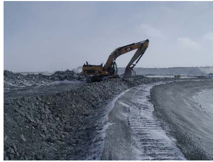
CD-1851 (2018-05-13), looking S from Sta. 0+910/-18 m. Excavation of the LLDPE geomembrane crest anchoring trench from Sta. 40+730 m to 0+830 m.
