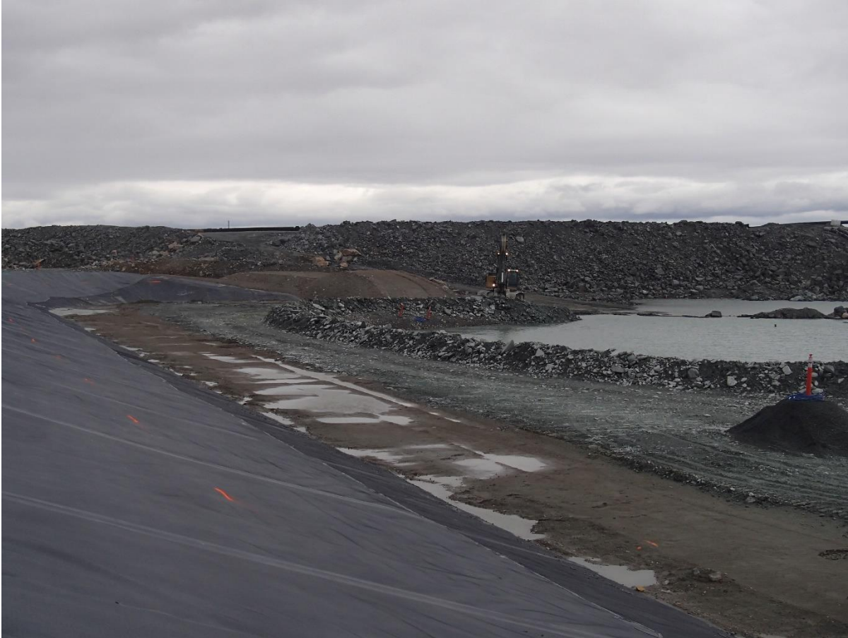
Photograph SD3-319: From Sta. 20+740/-31 m, looking SE. Placement of IV rockfill in the water up to El. 142m with an excavator from Sta. 20+730 m to 20+610 m, at the bottom of the upstream slope of SD3 to widen the rockfill layer and allow access to the erosion protection.
