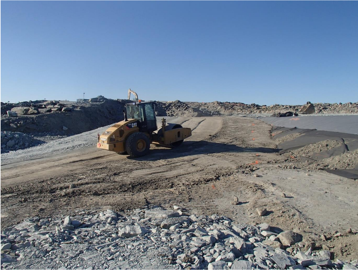
Photograph SD3-340: From Sta. 20+750/-40 m, looking S. Compaction of the third 0.5 m thick lift of compacted sieved till on the upstream toe liner tie-in with an excavator from Sta. 20+760 m to 20+820 m.
