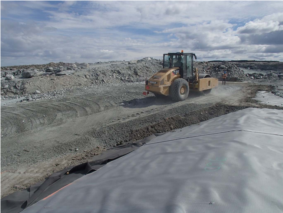
Photograph SD3-349: From Sta. 20+765/-29 m, looking SE. Compaction of the 0.5 m thick lift of fine filter on the top of the upstream toe liner tie-in with a 10 tonne smooth-drum compactor with vibration (4 passes) from Sta. 20+777 m to 20+807 m.
