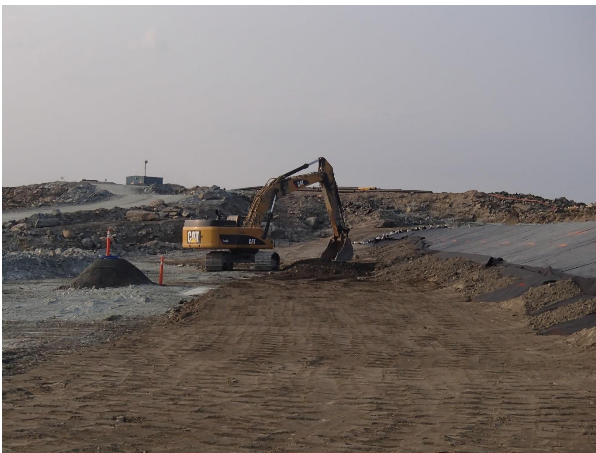
Photograph SD3-324: From Sta. 20+680/-39m, looking S. Placement of a 0.5 m thick lift of low quality till (0-150 mm) from El. 142 m to 142.5 m from Sta. 20+715 m to 20+760 m.
