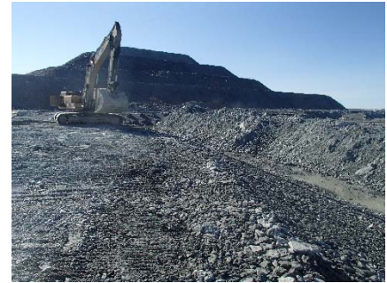
NCIS-051 (2018-06-27), looking SE from Sta. 2+630/-34 m. Placement of a 0.5 m thick lift of coarse filter in the upstream slope from El. 150 m to 152 m with an excavator from Sta. 2+640 m to 2+815 m.
