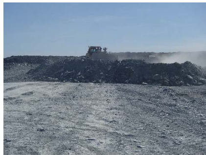
NCIS-098 (2018-07-19), looking E from Sta. 2+040/-9 m (approx.). Placement of a 2 m thick (approx.) lift of UM rockfill from El. 152 m to El. 154 m (approx.) with a dozer from Sta. 2+103 m to 1+984 m (+7 m to -22 m). The material is of good quality and is well graded.
