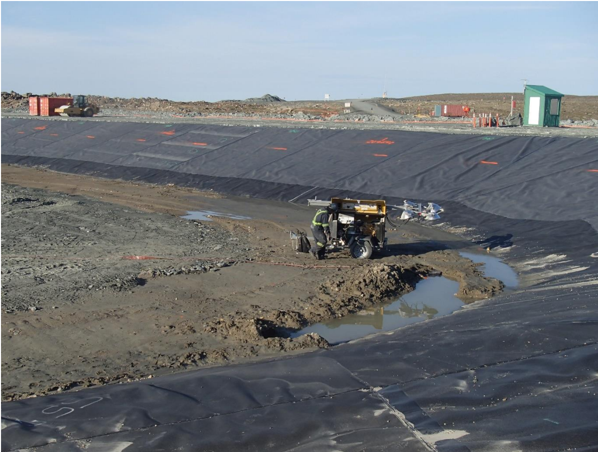
Photograph SD3-321: From Sta. 20+610/-56 m, looking SW. Water ponding at El. 142m on the compacted sieved till layer of the upstream toe liner tie-in at approx. Sta. 20+620 m to 20+630 m was pumped.
