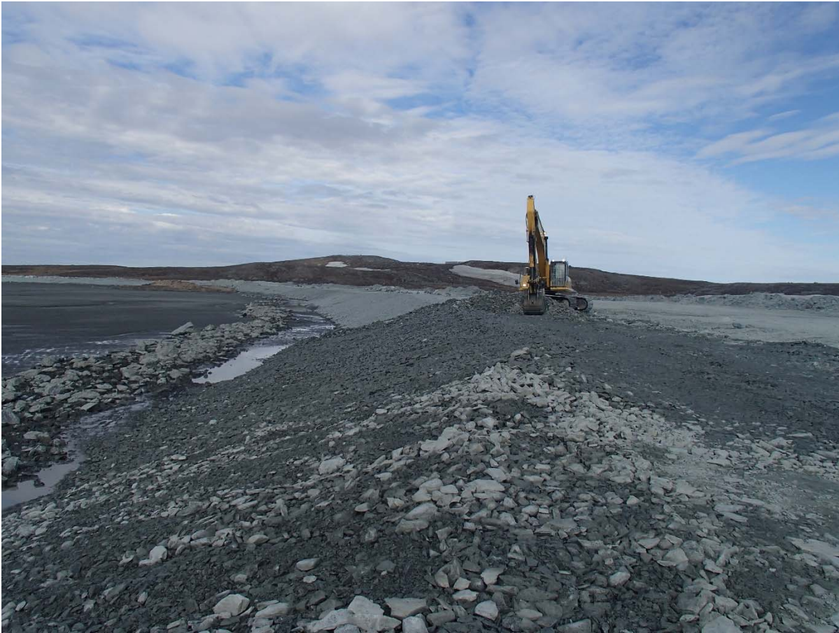
Photograph NCIS-030: From Sta. 2+140/-29 m (approx.), looking W. Placement of a 0.5 m thick lift of coarse filter in the upstream slope from El. 150 m to 152 m with an excavator from Sta. 2+105 m to 1+930 m. Notice the presence of water ponding at the bottom of the slope.
