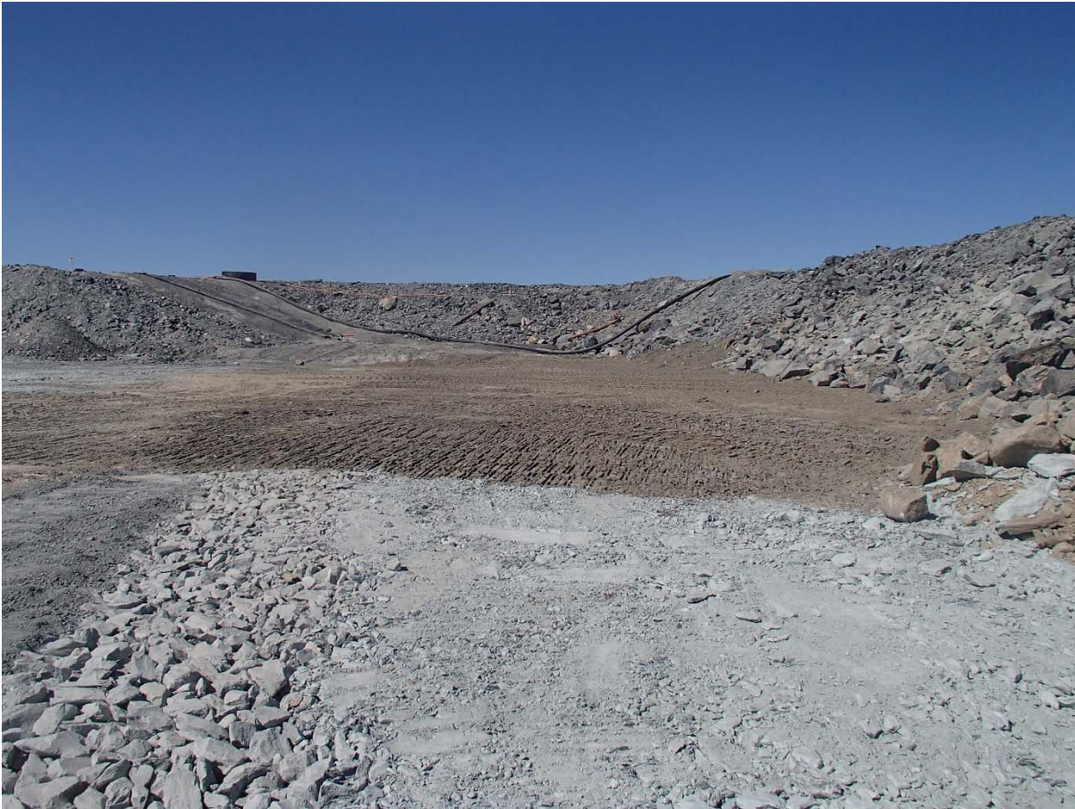
Photograph SD3-343: From Sta. 20+590/-40 m, looking NW. View of the depression between SD2 and SD3 backfilled with low quality till up to El. 145 m.
