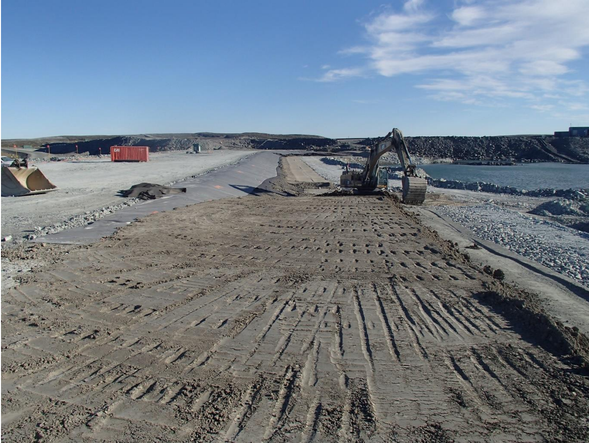
Photograph SD3-335: From Sta. 20+815/-27 m, looking N. Placement of a third 0.5 m thick lift of compacted sieved till on the upstream toe liner tie-in with an excavator from Sta. 20+760 m to 20+810 m.
