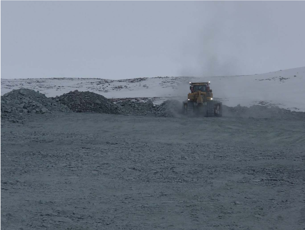
Photograph NCIS-011: From Sta. 2+000 m (approx.), looking SW. Placement a 2 m thick (approx.) lift of UM rockfill from El. 150 m to El. 152 m (approx.) with a dozer from Sta. 1+880 m to 1+767 m (o.s. unavailable).
