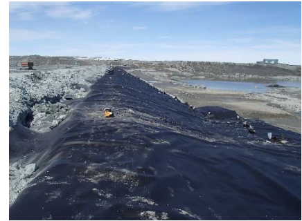
SD3-311 (2018-06-07), looking N from Sta. 20+810/-26 m. Installation of the LLDPE liner on the upstream slope 3H:1V between El. 143 m and 145 m from Sta. 20+630 m to 20+800 m (panel numbers 939 to 964).
