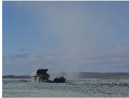
NCIS-059 (2018-06-29), looking S from Sta. 1+330/-34 m. Placement of a 1.5 to 2 m thick (approx.) lift of UM rockfill from El. 148 m to El. 150 m (approx.) with a dozer from Sta. 1+120 m to 1+100 m (-96 m to -60 m). The material is of good quality and is well graded.
