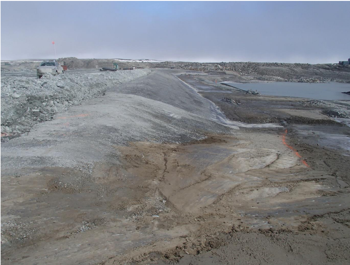
Photograph SD3-307: From Sta. 20+800/-25 m, looking N. View of the liner bedding ready for geosynthetics installation.
