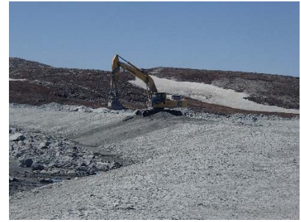
NCIS-039 (2018-06-23), looking W from Sta. 2+200/-24 m. Placement of a 0.5 m thick lift of fine filter over the coarse filter in the upstream slope from El. 150 m to 152 m with an excavator from Sta. 2+460 m to 2+475 m and from Sta. 2+065 m to 1+980 m.
