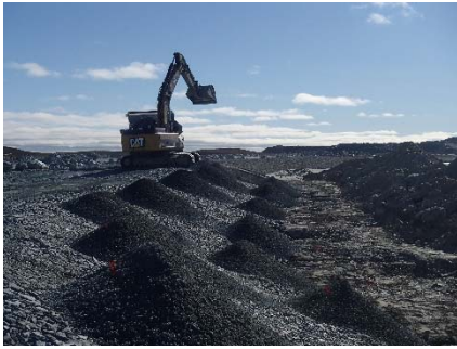
NCIS-055 (2018-06-28), looking NE from Sta. 1+730/-42 m. Placement of a 0.5 m thick lift of fine filter over the coarse filter in the upstream slope from El. 150 m to 152 m with an excavator from Sta. 1+820 m to 1+595 m.
