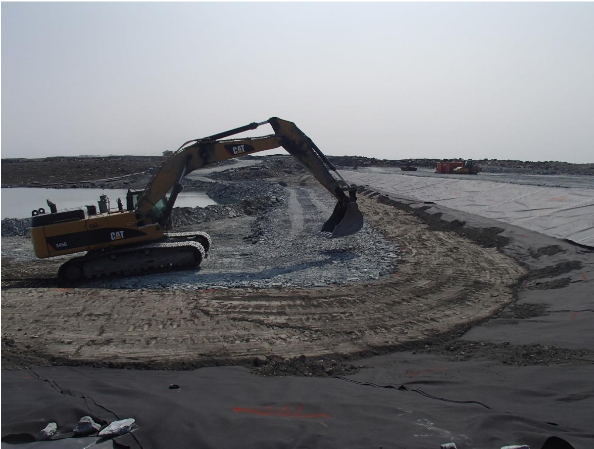
Photograph SD3-325: From Sta. 20+610/-43 m, looking S. Placement of a first 0.5 m thick lift of fine rockfill (0-500 mm) upstream of the low quality till from El. 142 m to 142.5 m from Sta. 20+610 m to 20+760 m.
