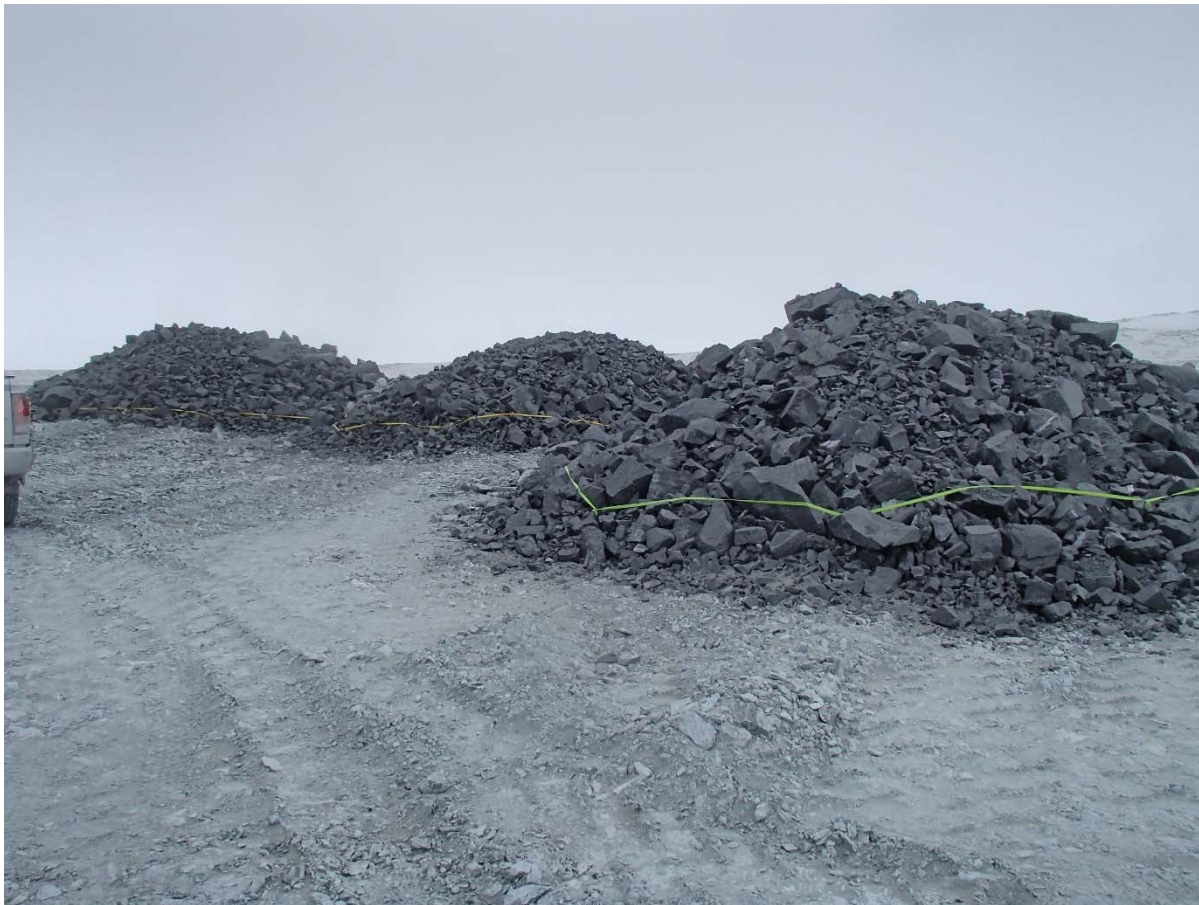
Photograph NCIS-016: From Sta. 1+750 m (approx.), looking SE. View of the Iron Formation rockfill (PAG material) piles on the North Cell Internal Structure to be cleaned from the structure embankment.
