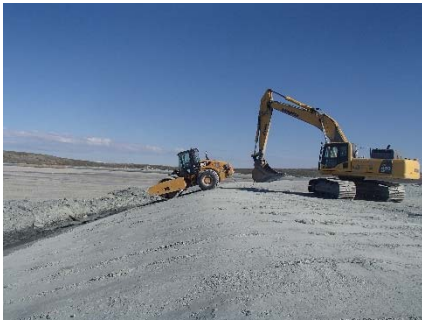
NCIS-112 (2018-07-24), looking N from Sta. 2+610/-29 m (approx.). Compaction of the 0.5 m lift (approx.) of coarse filter between El. 152 m and 154 m with a 10-tonne smooth-drum compactor with vibration (4 passes) in the upstream slope from Sta. 2+080 m to 2+000 m.
