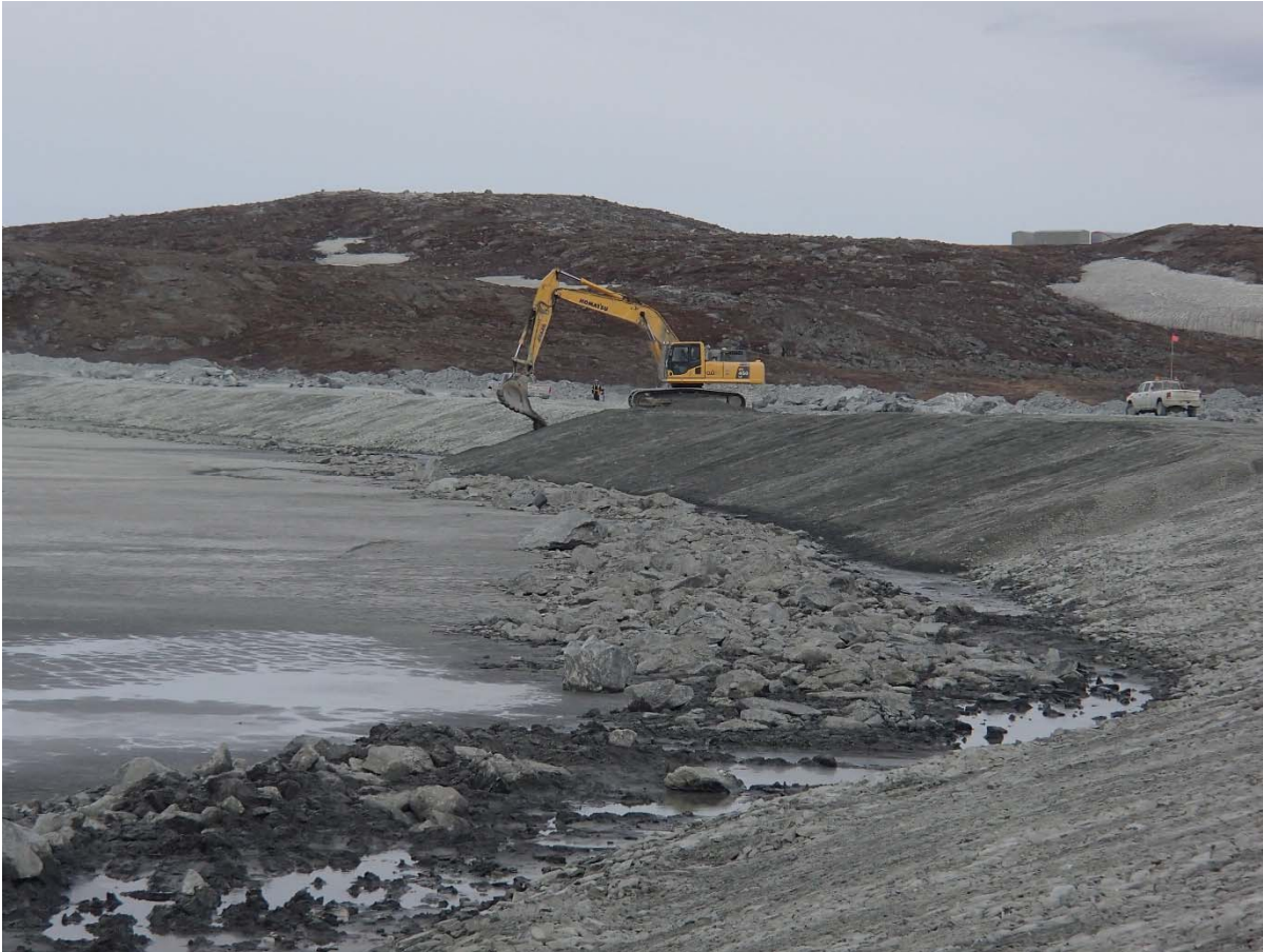
Photograph NCIS-040: From Sta. 2+185/-25 m (approx.), looking W. Placement of a 0.5 m thick lift of fine filter over the coarse filter in the upstream slope from El. 150 m to 152 m with an excavator from Sta. 2+305 m to 2+460 m and from Sta. 1+980 m to 1+835 m.
