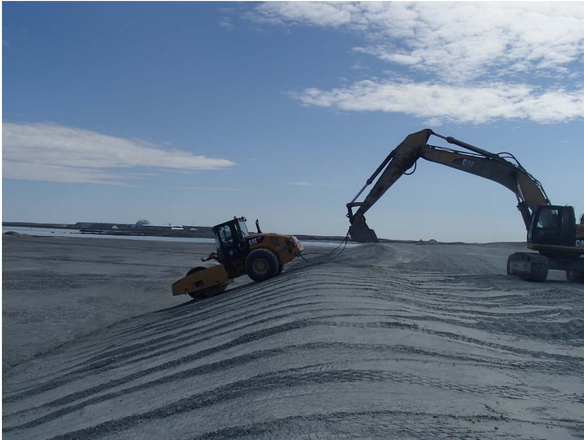
Photograph NCIS-107: From Sta. 1+380/-38 m (approx.), looking S. Compaction of the 0.5 m lift (approx.) of fine filter between El. 150 m and 152 m with a 10-tonne smooth-drum compactor with vibration (4 passes) in the upstream slope from Sta. 1+251 m to 1+1+660 m.
