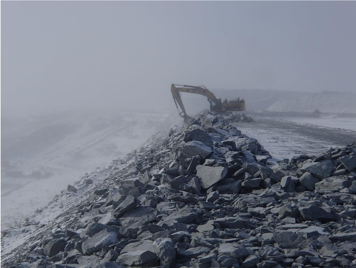
Photograph CD-1825: From Sta 0+430/+9 m, looking S. Profiling of the downstream slope (1.5H:1V) from El. 143 to 145 m with an excavator between Sta. 0+330 m and 0+440 m and between Sta. 0+530 m and 0+745 m.
