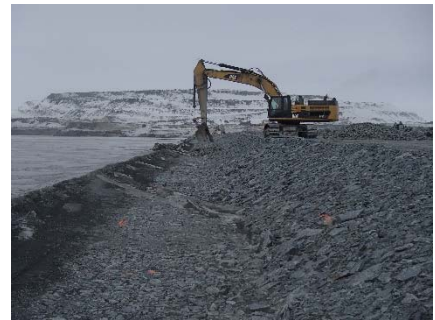
CD-1837 (2018-05-08), looking N from Sta. 0+940/-25 m. Placement of a second 0.5 m thick lift of coarse filter from El. 143.5 m to 144 m with an excavator from Sta. 0+290 m to 0+500 and from Sta. 0+835 m to 0+930 m.
