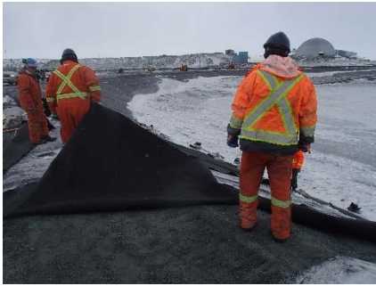
CD-1868 (2018-05-27), looking S from Sta. 0+915/-24 m. Removal of the wet geotextile in place from Sta. 0+935 m to 0+900 m.
