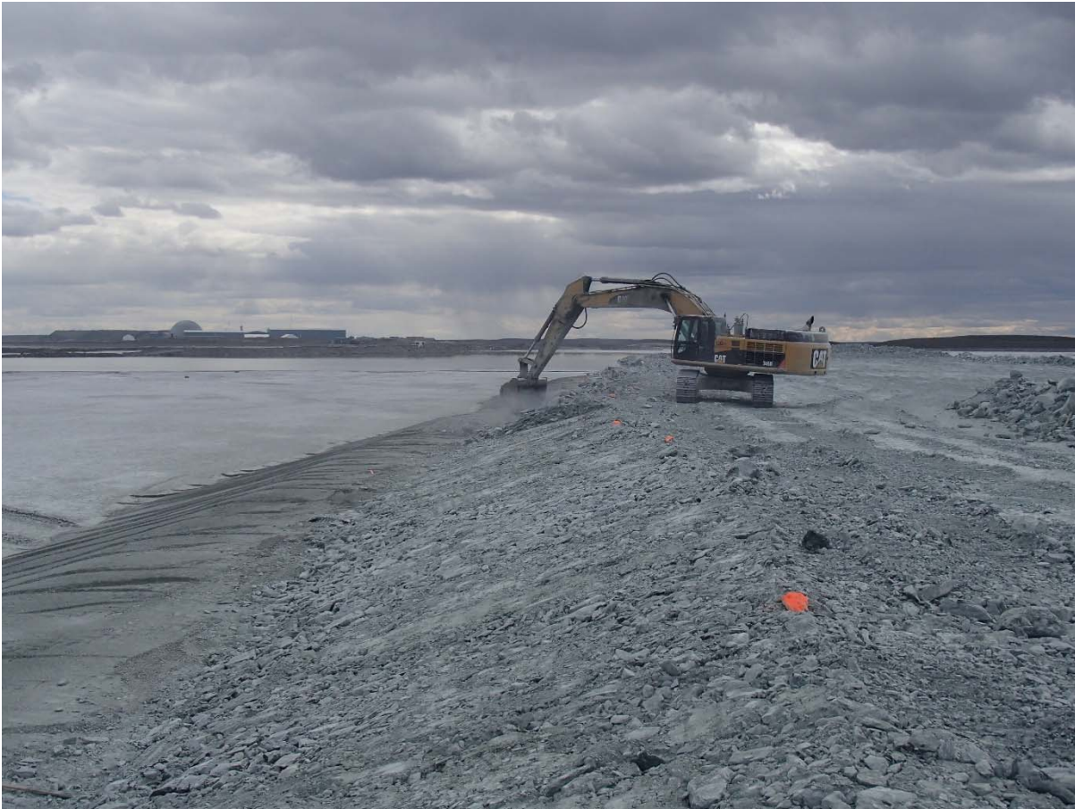
Photograph NCIS-077: From Sta. 1+310/-32 m (approx.), looking S. Profiling of the upstream slope (3H:1V) from El. 150 to 152 m with an excavator from Sta. 1+300 m to 1+175 m and from 3+070 m to 3+160 m.
