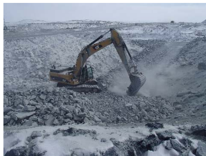
CD-1812 (2018-04-30), looking SE from Sta. 0+985/-11 m. Placement of intermediate volcanic (IV) rockfill on the existing downstream slope up to approx. El. 140 m, from approx. Sta. 0+985 to 40+780 m.
