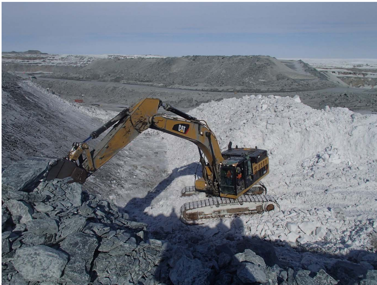
Photograph CD-1803: From Sta. 40+750/27 m looking NE. Removal of snow to expose the foundation bedrock with an excavator between approx. Sta. 40+780 and 40+800 m (o.s. 7 to 10 m).
