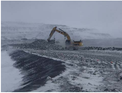
CD-1814 (2018-05-01), looking NE from Sta. 0+970/-10 m. Placement of intermediate volcanic (IV) rockfill around the instruments at approx. Sta. 0+830 m with the excavator.
