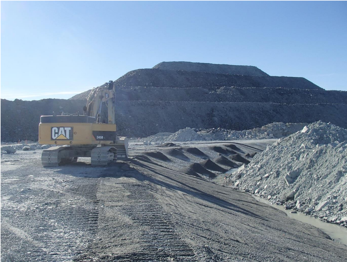
Photograph NCIS-071: From Sta. 2+670/-28 m (approx.), looking SE. Placement of a 0.5 m thick lift of fine filter over the coarse filter in the upstream slope from El. 150 m to 152 m with an excavator from Sta. 1+550 m to 1+320 m and 1+630 m to 1+610 m.
