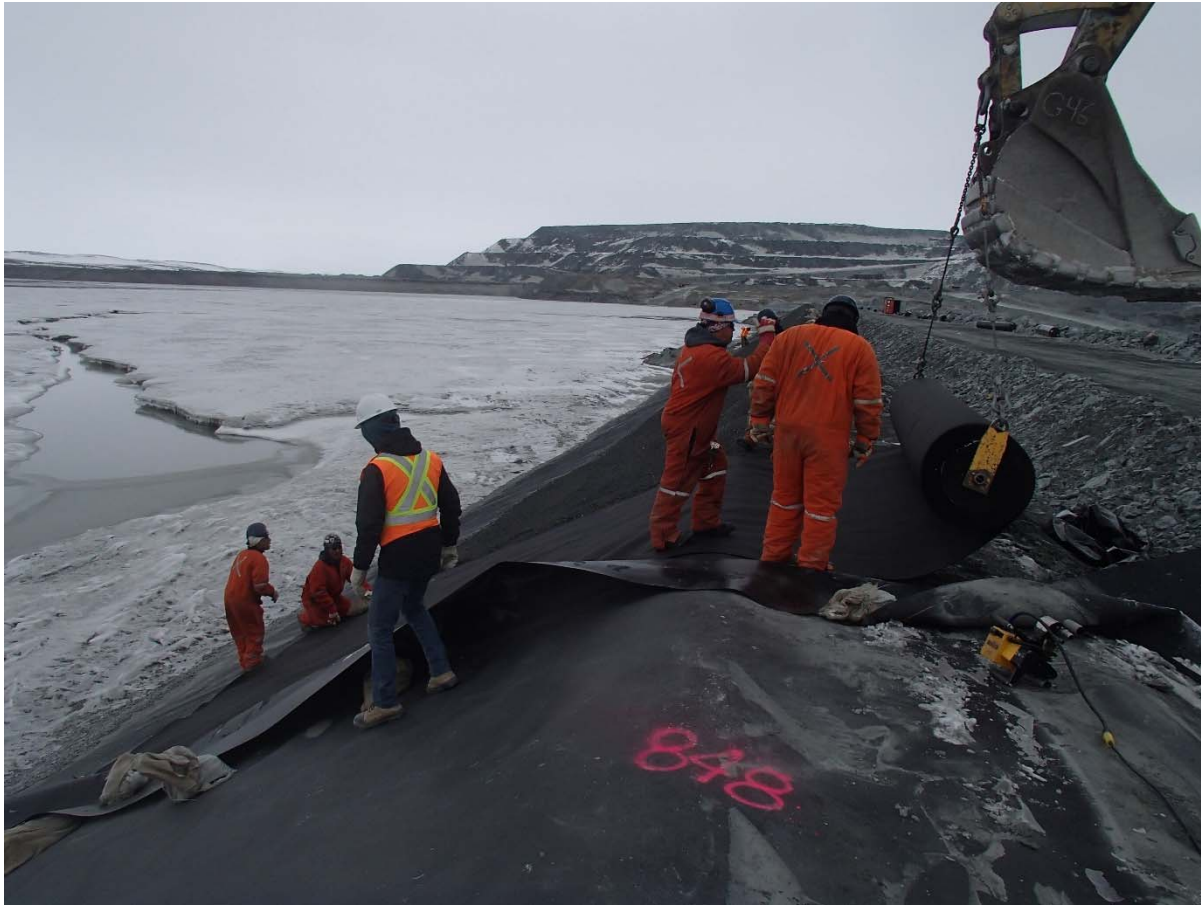
Photograph CD-1877: From Sta. 0+745/-26 m, looking N. Installation of the geotextile on the upstream slope 2H:1V between El. 143 m and 145 m from Sta. 0+740 m to 0+610 m.
