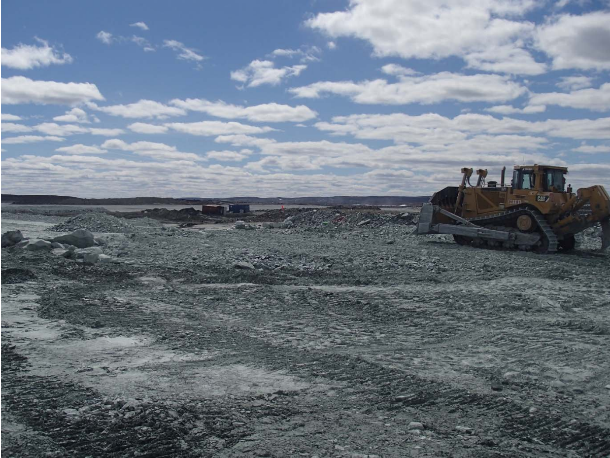
Photograph NCIS-060: From Sta. 1+365/-35 m (approx.), looking SW. Placement of a 2 m thick (approx.) lift of UM rockfill from El. 150 m to El. 152 m (approx.) with a dozer from Sta. 1+340 m to 1+320 m (-19 m to +16 m). The material is of good quality and is well graded.
