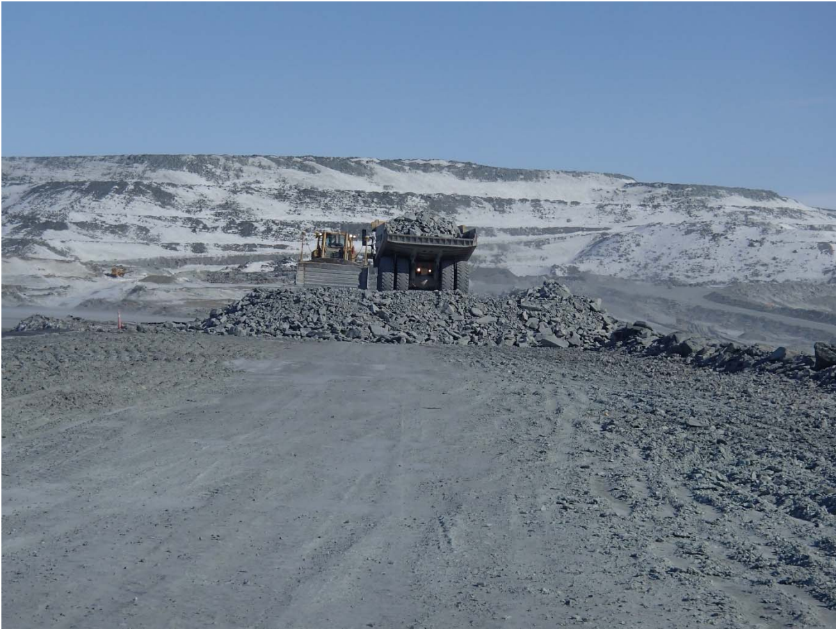
Photograph CD-1802: From Sta. 0+770/-16 m looking N. Placement of a 2 m thick (approx.) lift of intermediate volcanic (IV) rockfill from El. 143 m to El. 145 m from approx. Sta. 0+525 to 0+710 m (o.s. -28 to -18 m).
