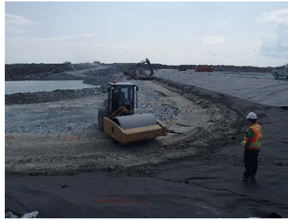
SD3-328 (2018-07-11), looking N from Sta. 20+820/-34 m. Compaction perpendicular to the longitudinal axis of Saddle Dam 3 of the 0.5 m lift of low quality till (0-150 mm) at El. 142.5 m with a 10-tonne smooth-drum compactor without vibration (4 passes) from Sta. 20+615m to 20+635 m.
