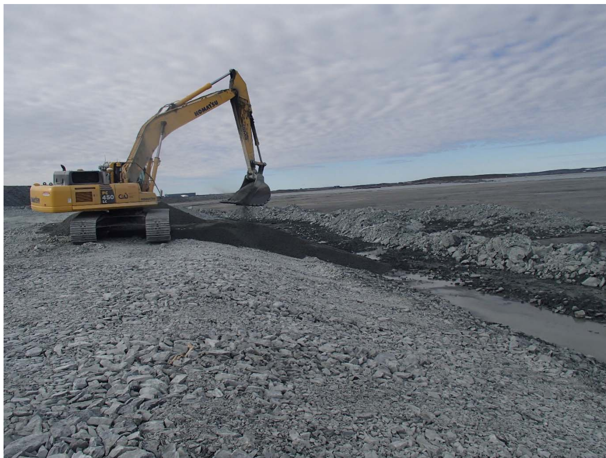
Photograph NCIS-036: From Sta. 1+900/-21 m (approx.), looking SE. Placement of a 0.5 m thick lift of fine filter over the coarse filter in the upstream slope from El. 150 m to 152 m with an excavator from Sta. 2+542 m to 2+475 m.
