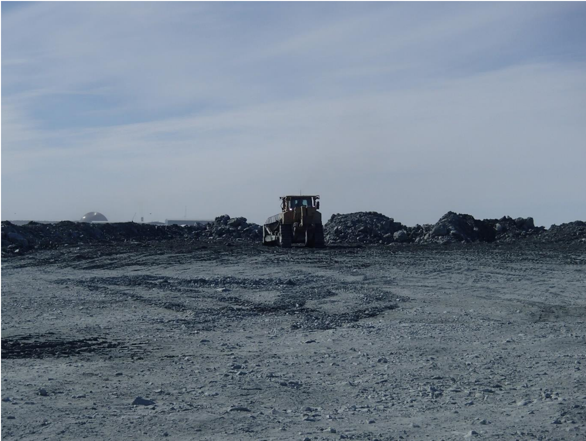
Photograph NCIS-026: From Sta. 1+440/+2 m, looking S. Placement of a 2 m thick (approx.) lift of UM rockfill from El. 150 m to El. 152 m (approx.) with a dozer from Sta. 1+390 m to 1+365 m (o.s. +10 m to -29 m).
