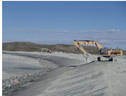
NCIS-113 (2018-07-24), looking SW from Sta. 2+220/-26 m (approx.). Profiling of the upstream slope (3H:1V) from El. 152 to 154 m with an excavator from Sta. 2+000 m to 1+185 m and placement of a 0.5 m thick lift of fine filter in the upstream slope from El. 152 m to 154 m with an excavator from Sta. 2+300 m to 2+090 m.
