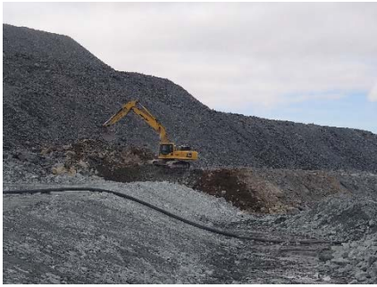
NCIS-046 (2018-06-26), looking SE from Sta. 2+680/-18 m. Removal of till material mixed with the UM rockfill of the capping (about 1 to 2 m thick along the slope) with an excavator from Sta. 2+760 m to 2+850 m (o.s. -35 to -17 m).
