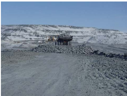
CD-1802 (2018-04-27), looking N from Sta. 0+770/-16 m. Placement a 2 m thick (approx.) lift of intermediate volcanic (IV) rockfill from El. 143 m to El. 145 m from approx. Sta. 0+625 to 0+710 m (o.s. -28 to -18 m).
