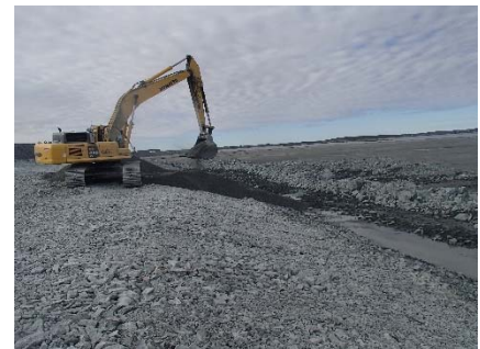
NCIS-036 (2018-06-22), looking SE from Sta. 1+900/-21 m. Placement of a 0.5 m thick lift of fine filter over the coarse filter in the upstream slope from El. 150 m to 152 m with an excavator from Sta. 2+542 m to 2+475 m.
