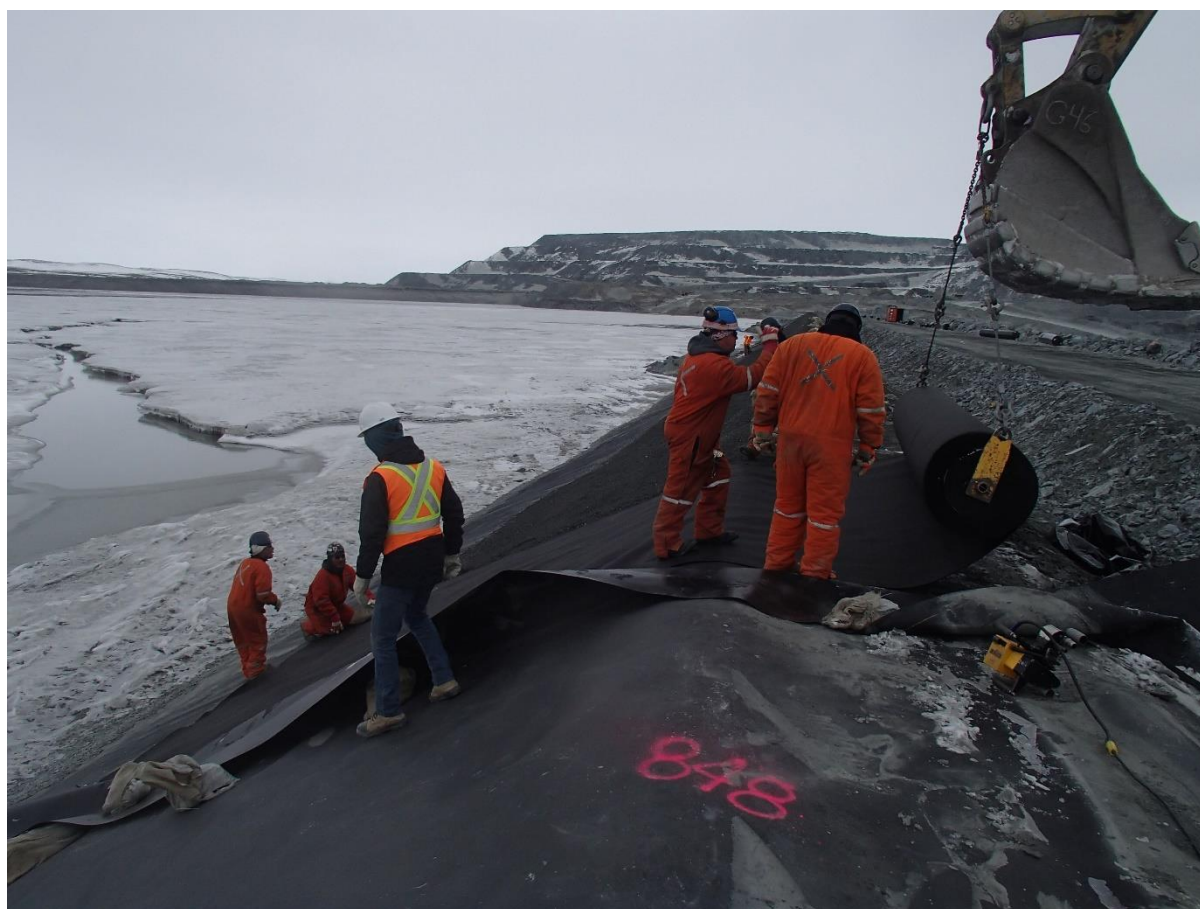
Photograph CD-1877: From Sta. 0+745/-26 m, looking N. Installation of the geotextile on the upstream slope 2H:1V between El. 143 m and 145 m from Sta. 0+740 m to 0+610 m.
