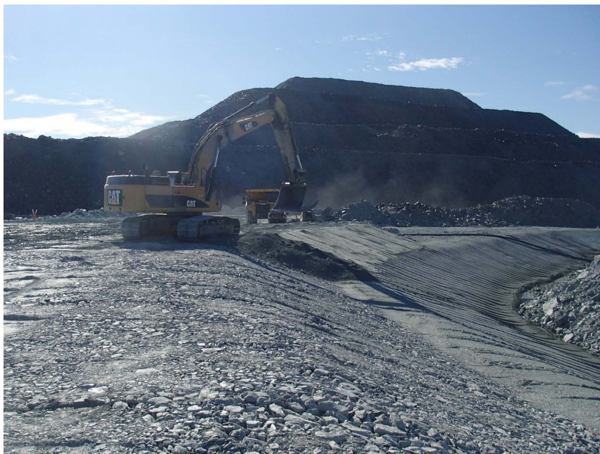
Photograph NCIS-104: From Sta. 2+650/-23 m (approx.), looking SE. Placement of a 0.5 m thick lift of fine filter in the upstream slope from El. 152 m to 154 m with an excavator from Sta. 2+710 m to 2+445 m.
