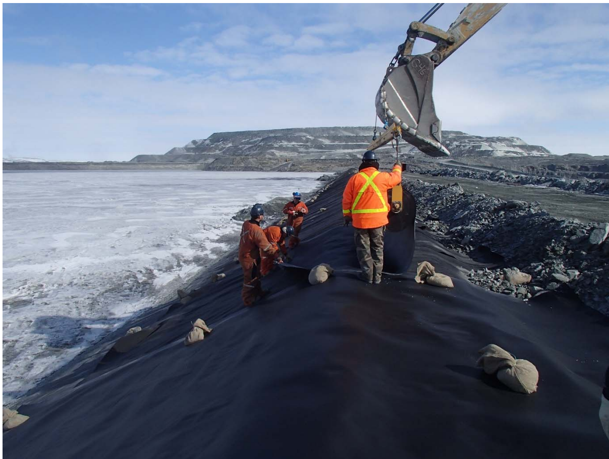
Photograph CD-1878: From Sta. 0+720/-24 m, looking N. Installation of the LLDPE liner on the upstream slope 2H:1V between El. 143 m and 145 m from Sta. 0+740 m to 0+610 m (panel numbers 849 to 867).
