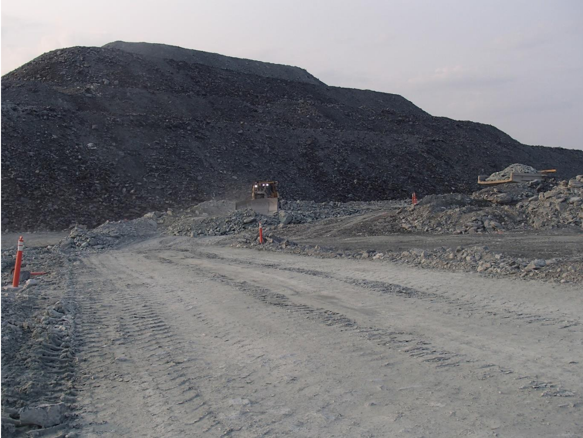
Photograph NCIS-086: From Sta 2+750/+14 m (approx.), looking E. Placement of a 2 m thick (approx.) lift of UM rockfill from El. 152 m to El. 154 m (approx.) with a dozer from Sta. 2+780 m to 2+760 m (-60 m to -44 m).
