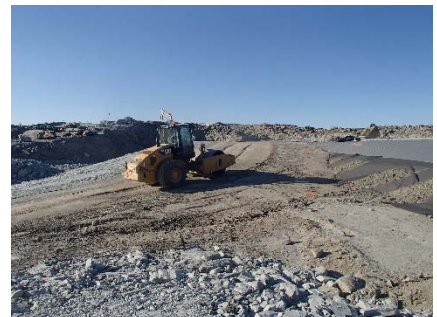
SD3-340 (2018-07-15), looking S from Sta. 20+750/-40 m. Compaction of the third 0.5 m thick lift of compacted sieved till on the upstream toe liner tie-in with an excavator from Sta. 20+760 m to 20+820 m.
