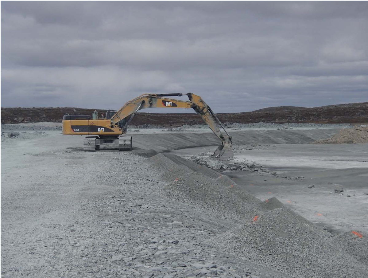
Photograph NCIS-062: From Sta. 1+525/-33 m (approx.), looking N. Placement of a 0.5 m thick lift of fine filter over the coarse filter in the upstream slope from El. 150 m to 152 m with an excavator from Sta. 1+330 m to 1+260 m and from Sta. 1+595 m to 1+550 m.
