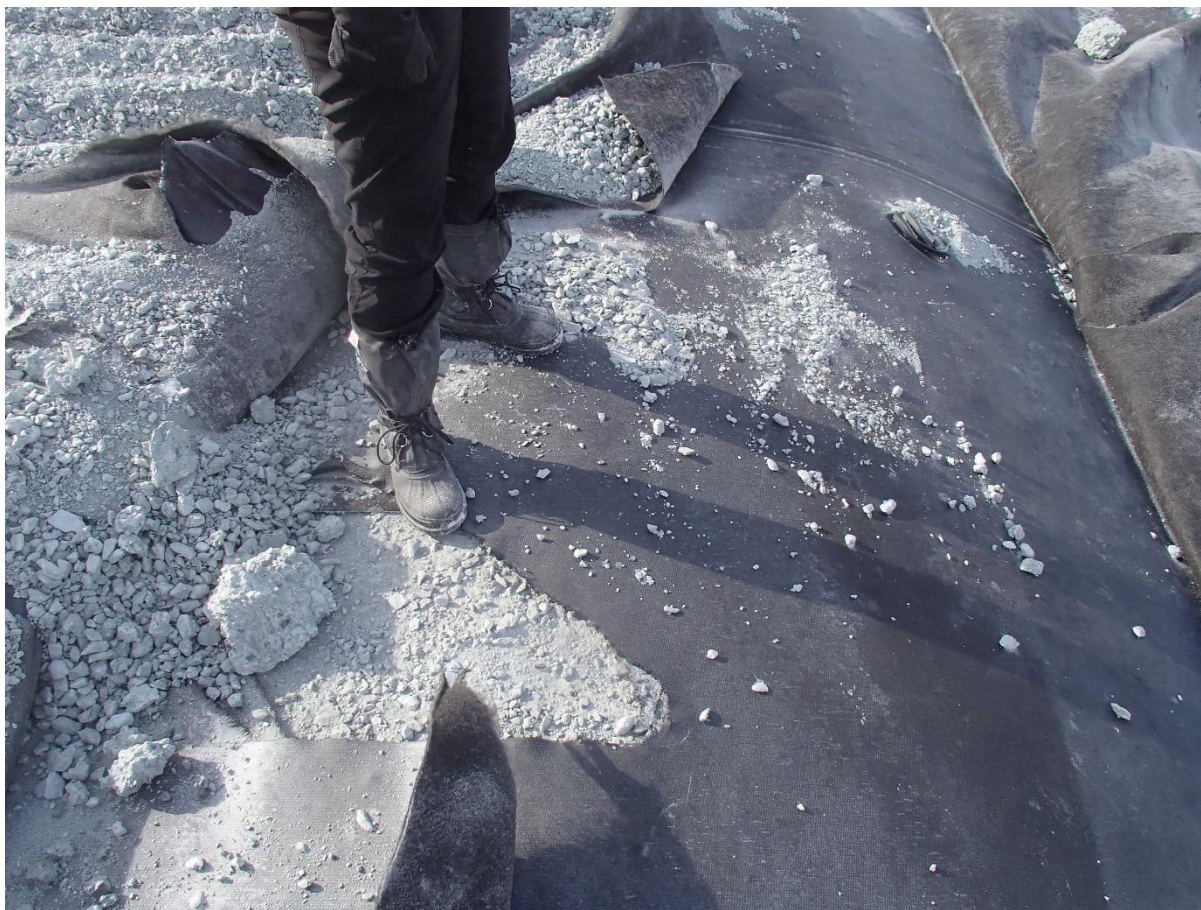
Photograph CD-1833: From Sta 0+390/-25 m, looking S. Damaged geomembrane near a deposition finger on Central Dike at Sta. 0+390 m.
