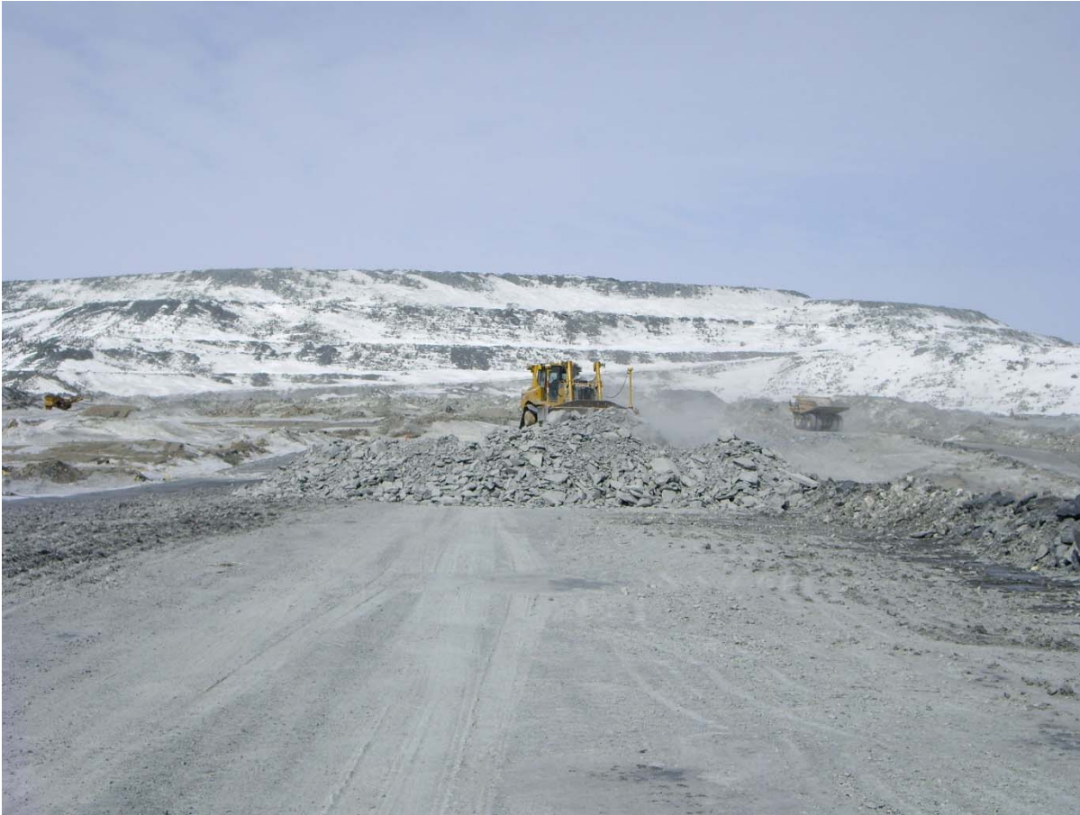
Photograph CD-1797: From Sta. 0+320/-20 m, looking N. Placement of a 2 m thick (approx.) lift of intermediate volcanic (IV) rockfill from El. 143 m to El. 145 m from 0+250 to 0+400 m (o.s. -28 to -18 m).
