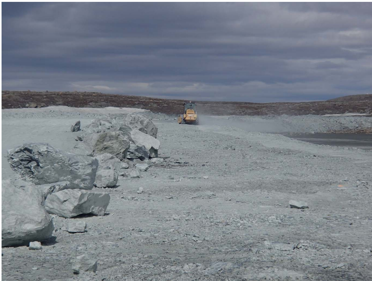
Photograph NCIS-032: From Sta. 1+400/-24 m (approx.), looking N. Compaction of the 2 m lift (approx.) of ultramafic (UM) rockfill at El. 152 m with a 10-tonne smooth-drum compactor with vibration (6 passes) between the haul truck traffic lane and the upstream slope from Sta. 1+660 to 1+380 m (offset -45 to -24 m).
