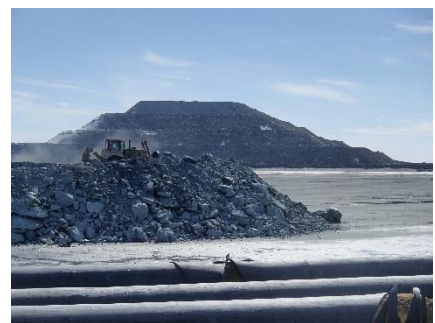
NCIS-027 (2018-06-07), looking E from Sta. 1+360/+67 m. Placement of a 2 m thick (approx.) lift of UM rockfill from El. 150 m to El. 152 m (approx.) with a dozer from Sta. 1+365 m to 1+360 m (+9 m to -28 m).
