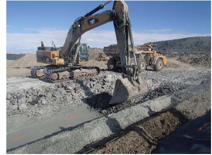
CD-1897 (2018-07-22), looking NW from Sta. 0+145/-30 m. Placement of a 0.5 m thick lift of coarse filter on the top of the fine filter on the top of the upstream toe liner tie-in and on the upstream slope with an excavator from Sta. 0+147 m to 0+177 m.
