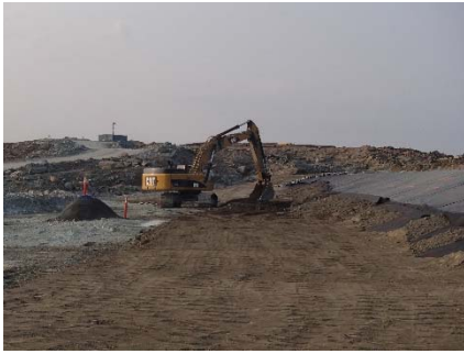
SD3-324 (2018-07-10), looking S from Sta. 20+680/-39 m. Placement of a 0.5 m thick lift of low quality till (0-150 mm) from El. 142 m to 142.5 m from Sta. 20+715 m to 20+760 m.
