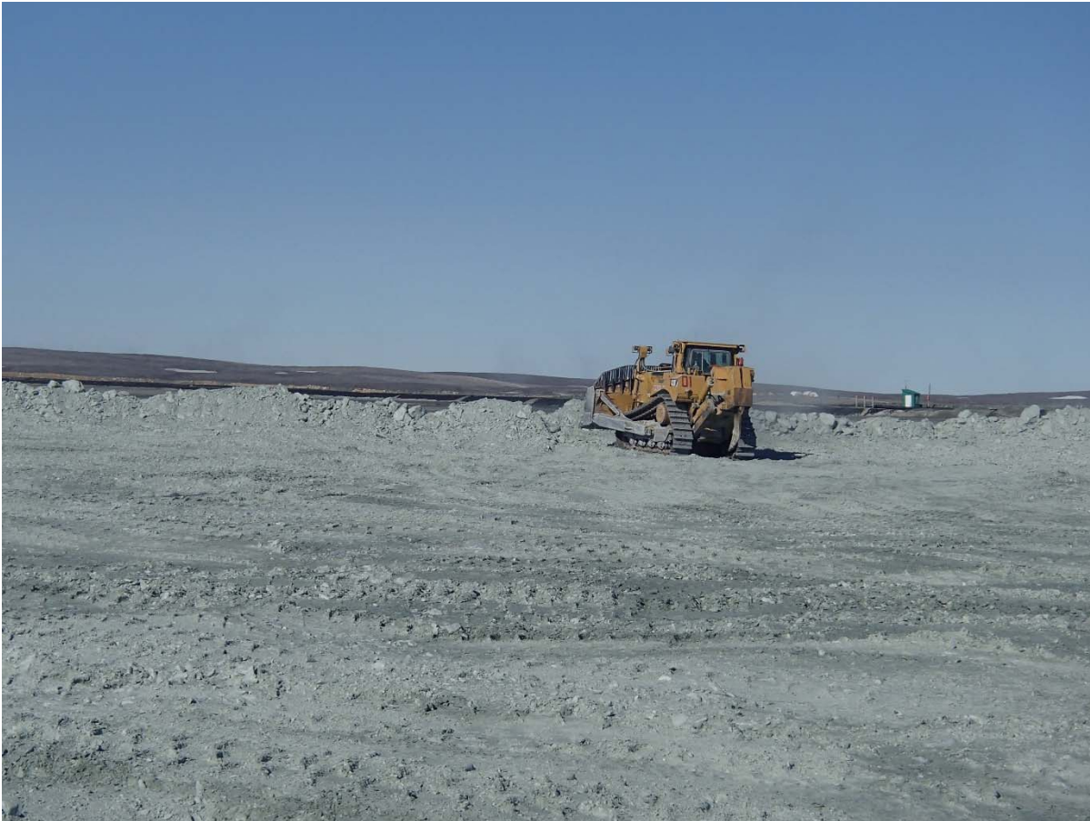
Photograph NCIS-052: From Sta. 1+120/-87 m (approx.), looking SW. Placement of a 1.5 to 2 m thick (approx.) lift of UM rockfill from El. 148 m to El. 150 m (approx.) with a dozer from Sta. 1+115 m to 1+100 m (-107 m to -45 m). The material is of good quality and is well graded.
