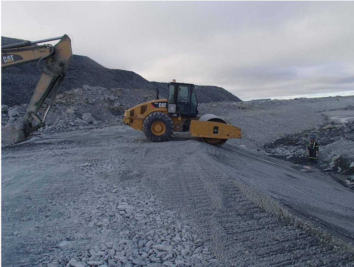
Photograph NCIS-074: From Sta. 2+750/-37 m (approx.), looking SE. Compaction of the 0.5 m lift (approx.) of fine filter between El. 150 m and 152 m with a 10-tonne smooth-drum compactor (4 passes) in the upstream slope from Sta. 2+810 m to 2+095 m. Vibration is used except for the first pass down the slope in order to stabilize the material and limit deformation of the lift.
