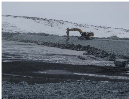
NCIS-017 (2018-05-24), looking SW from Sta. 2+290 m. Profiling of the upstream slope (3H:1V) from El. 150 to 152 m with an excavator from Sta. 2+138 m to 1+989 m.
