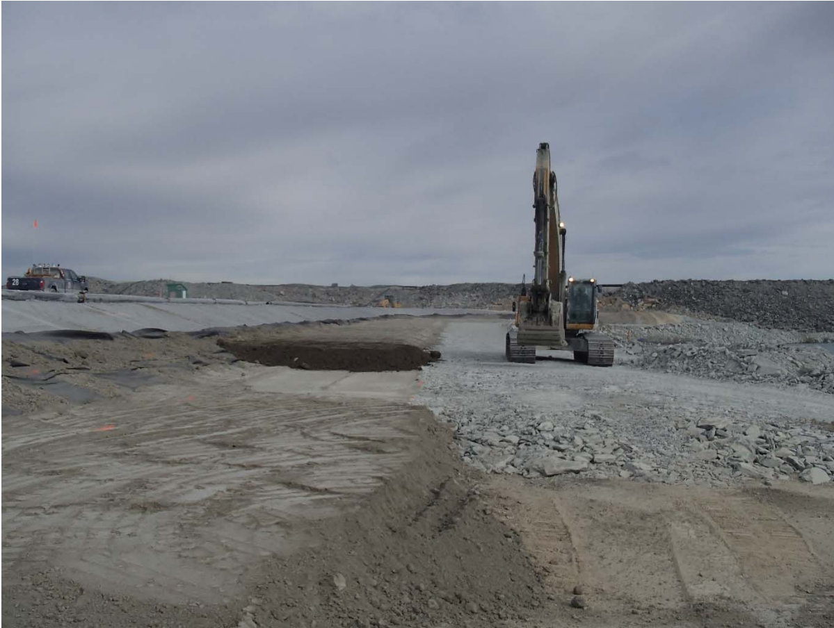
Photograph SD3-345: From Sta. 20+760/-42 m, looking NW. Placement of a fourth 0.5 m thick lift of low quality till (0-150 mm) from El. 143 m to 143.5 m from Sta. 20+619 m to 20+777 m.
