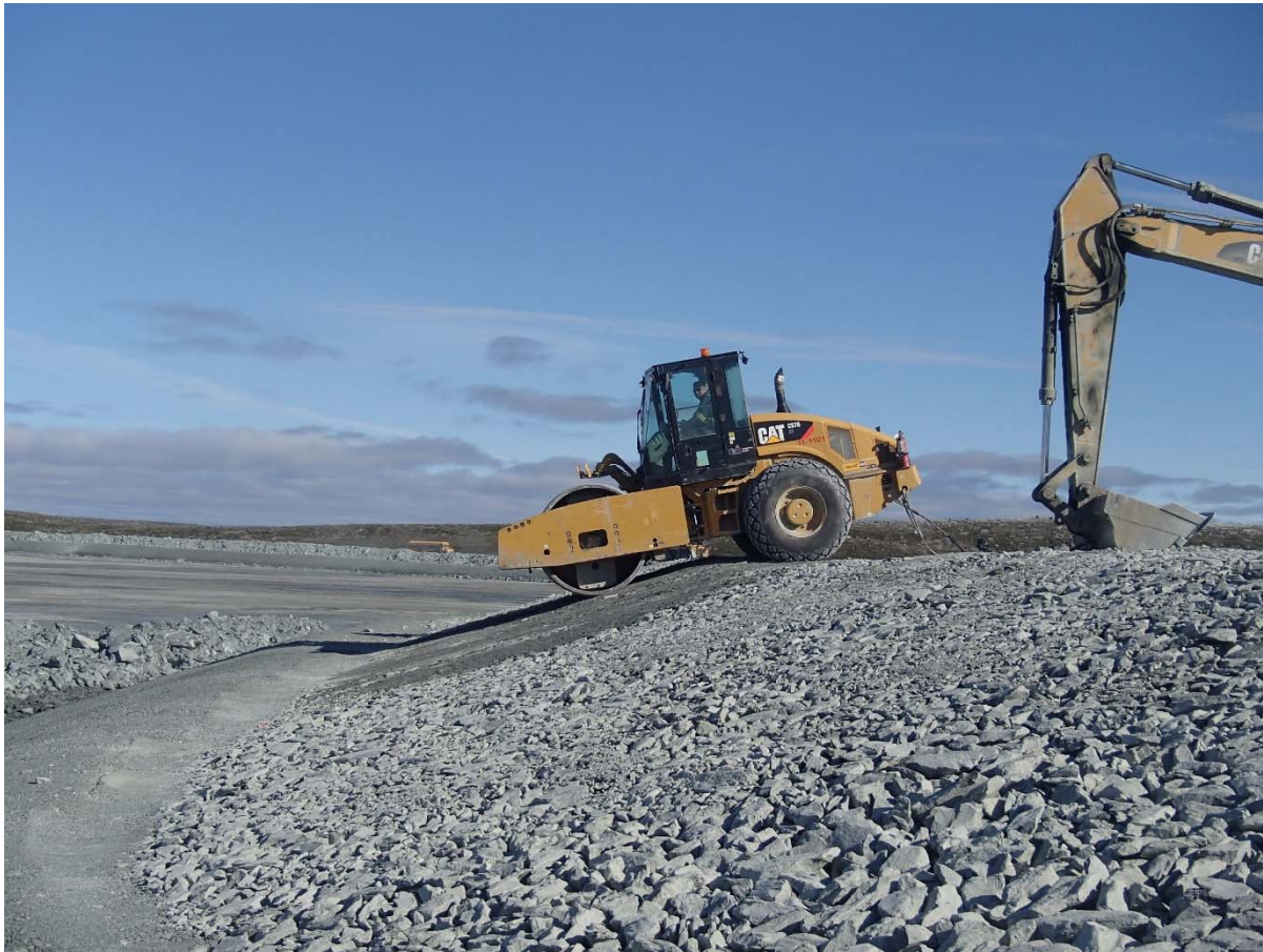
Photograph NCIS-105: From Sta. 2+630/-34 m (approx.), looking NW. Compaction of the 0.5 m lift (approx.) of coarse filter between El. 152 m and 154 m with a 10-tonne smooth-drum compactor with vibration (4 passes) in the upstream slope from Sta. 2+710 m to 2+411 m.
