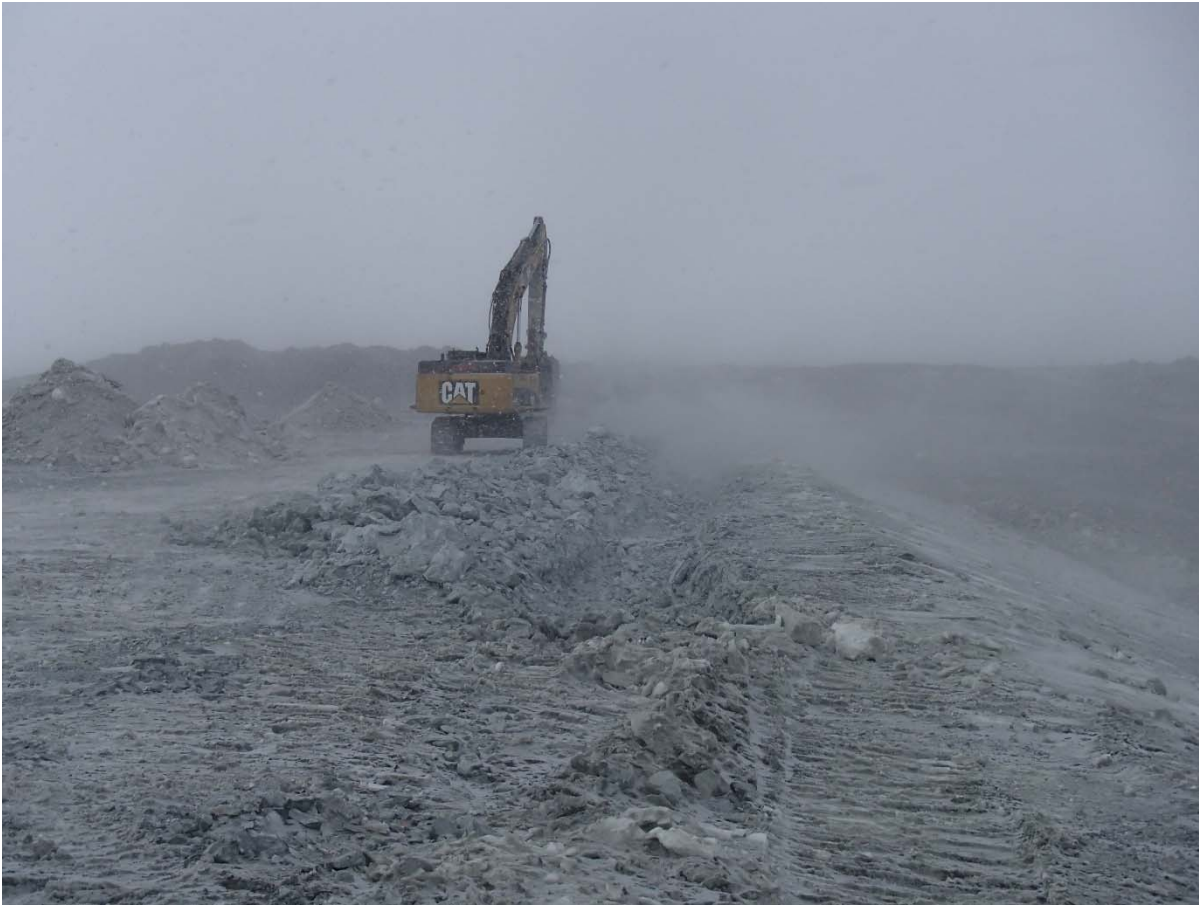
Photograph SD3-300: From Sta. 20+790/-33 m, looking NW. Excavation of the LLDPE geomembrane crest anchoring trench with an excavator from Sta. 20+675 m to 20+780 m.
