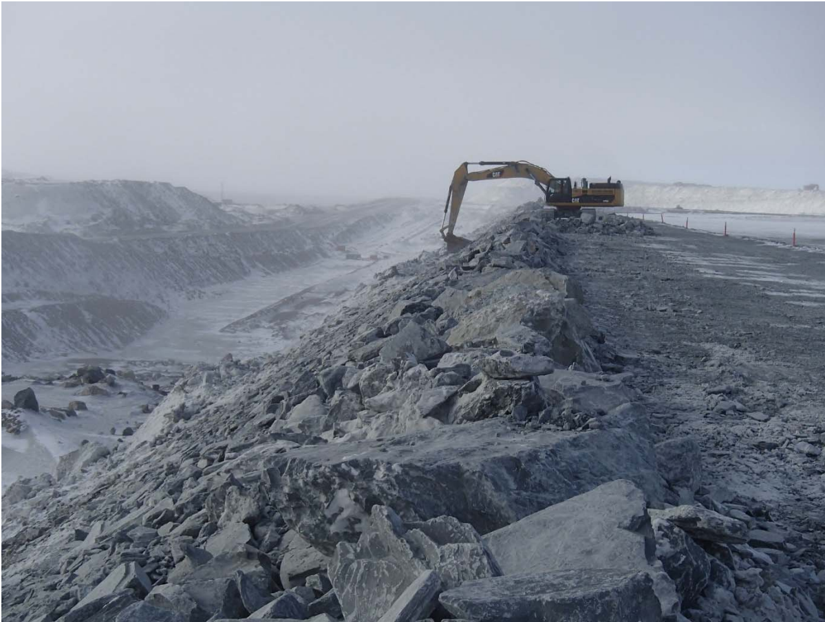
Photograph CD-1821: From Sta. 0+175/+3, looking S. Profiling of the downstream slope (1.5H:1V) from El. 143 to 145 m with an excavator between Sta. 0+250 m and 0+330 m.
