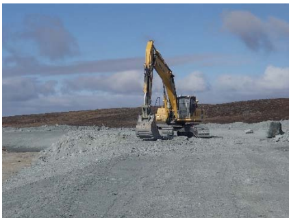
NCIS-034 (2018-06-21), looking W from Sta. 1+900/-21 m. Profiling of the upstream slope (3H:1V) from El. 150 to 152 m with an excavator from Sta. 1+860 m to 1+750 m.
