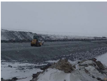
CD-1847 (2018-05-12), looking SE from Sta. 0+085/-48 m. Compaction of the fourth 0.5 m lift (approx.) of fine and coarse filters material at El. 145 m with a 10-tonne smooth-drum compactor with vibration (4 passes) from Sta 0+170 m to 0+930 m.
