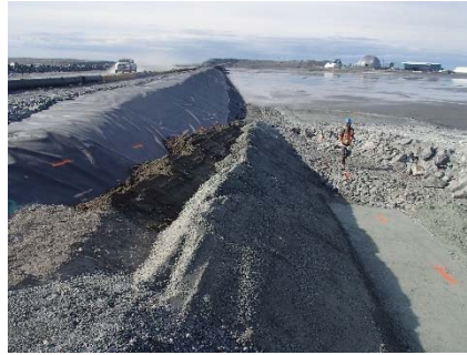
CD-1896 (2018-07-22), looking S from Sta. 0+140/-30 m. Placement of 0.5 m thick layers of compacted sieved till and fine filter on the upstream slope of Central Dike with an excavator from Sta. 0+147 m to 0+177 m.
