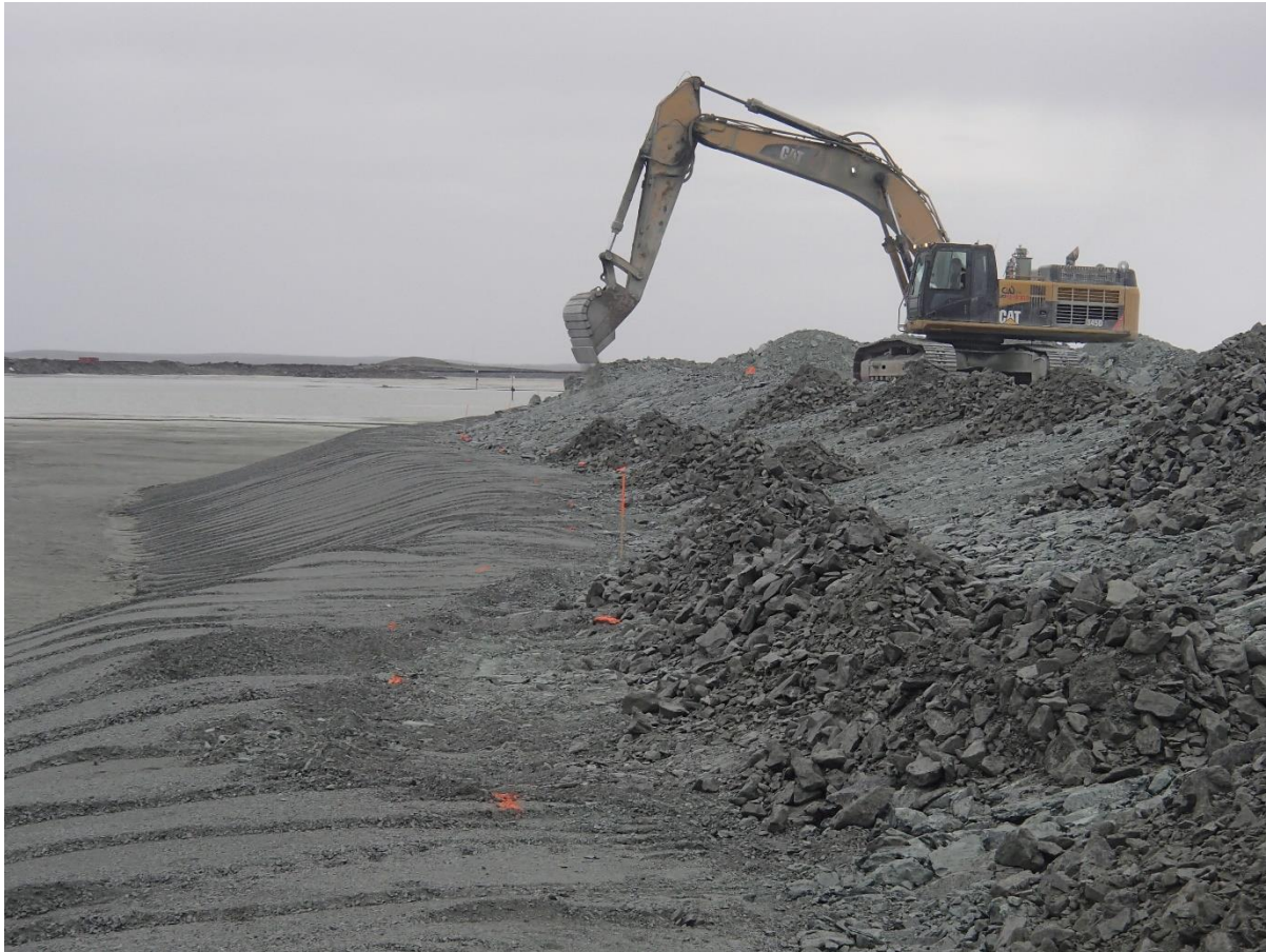
Photograph NCIS-079: From Sta. 1+280/-39 m (approx.), looking SW. Placement of a 0.5 m thick lift of coarse filter in the upstream slope from El. 150 m to 152 m with an excavator from Sta. 1+300 m to 1+200 m.
