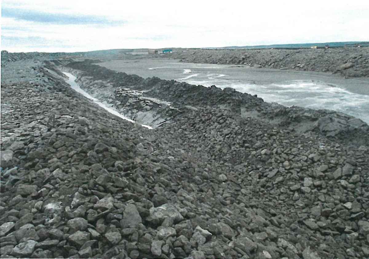
Photograph NCIS-138: From Sta. 1+365/+15 m (approx.), looking SW. Excavation of a 0.8 m (approx.) deep, 1 m wide shallow ditch in the tailings and placement of a 0.3 m thick (approx.) layer of till sieving reject material on the bottom and on the slopes of the ditch from Sta. 1+200 m to 1+100 m.
