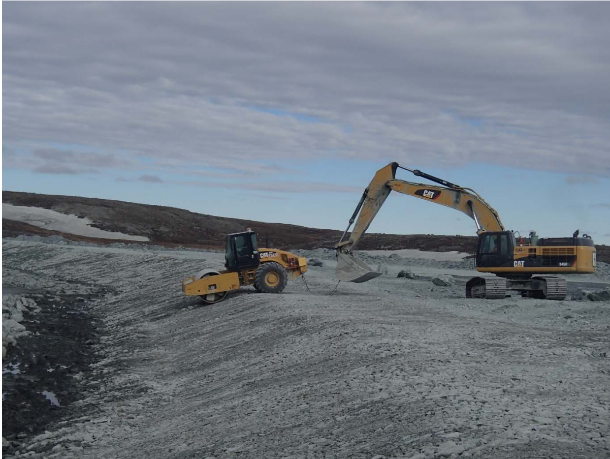
Photograph NCIS-037: From Sta. 1+550/-25 m (approx.), looking NW. Compaction of the 0.5 m lift (approx.) of coarse filter between El. 150 and 152 m with a 10-tonne smooth-drum compactor (4 passes) in the upstream slope from Sta. 2+450 to 1+805 m.
