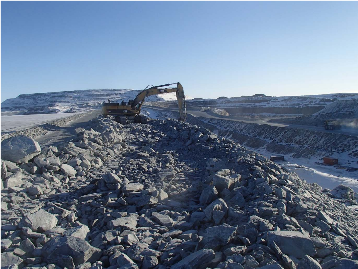
Photograph CD-1854: From Sta. 0+960/-13 m, looking N. Profiling of the downstream slope (1.5H:1V) from El. 143 to 145 m with an excavator between Sta. 0+940 m and 0+990 m.
