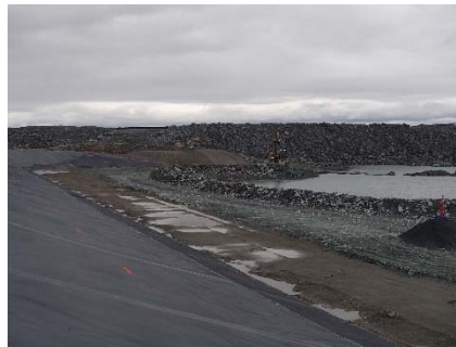
SD3-319 (2018-07-08), looking NE from Sta. 20+740/-31 m. Placement of IV rockfill in the water up to El. 142m with an excavator from Sta. 20+730 m to 20+610 m, at the bottom of the upstream slope of SD3 to widen the rockfill layer and allow access to the erosion protection.
