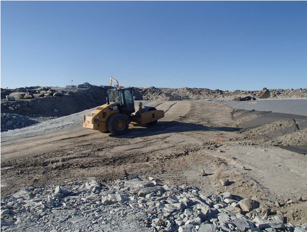
Photograph SD3-340: From Sta. 20+750/-40 m, looking S. Compaction of the third 0.5 m thick lift of compacted sieved till on the upstream toe liner tie-in with an excavator from Sta. 20+760 m to 20+820 m.
