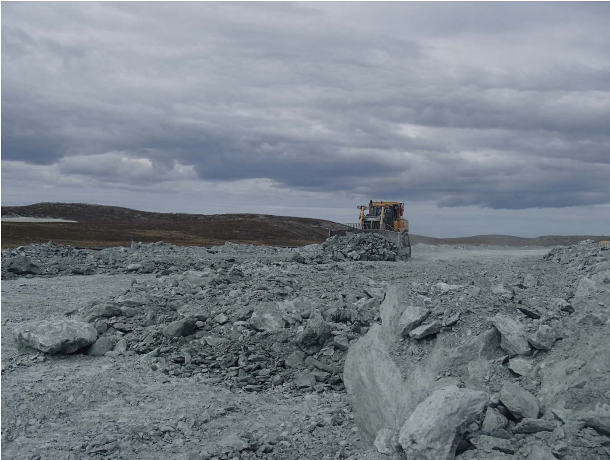
Photograph NCIS-069: From Sta. 1+180/-56 m (approx.), looking NW. Placement of a 2 m thick (approx.) lift of UM rockfill from El. 150 m to El. 152 m (approx.) with a dozer from Sta. 1+235 m to 1+160 m (-60 m to -44 m). The material is of good quality and is well graded.
