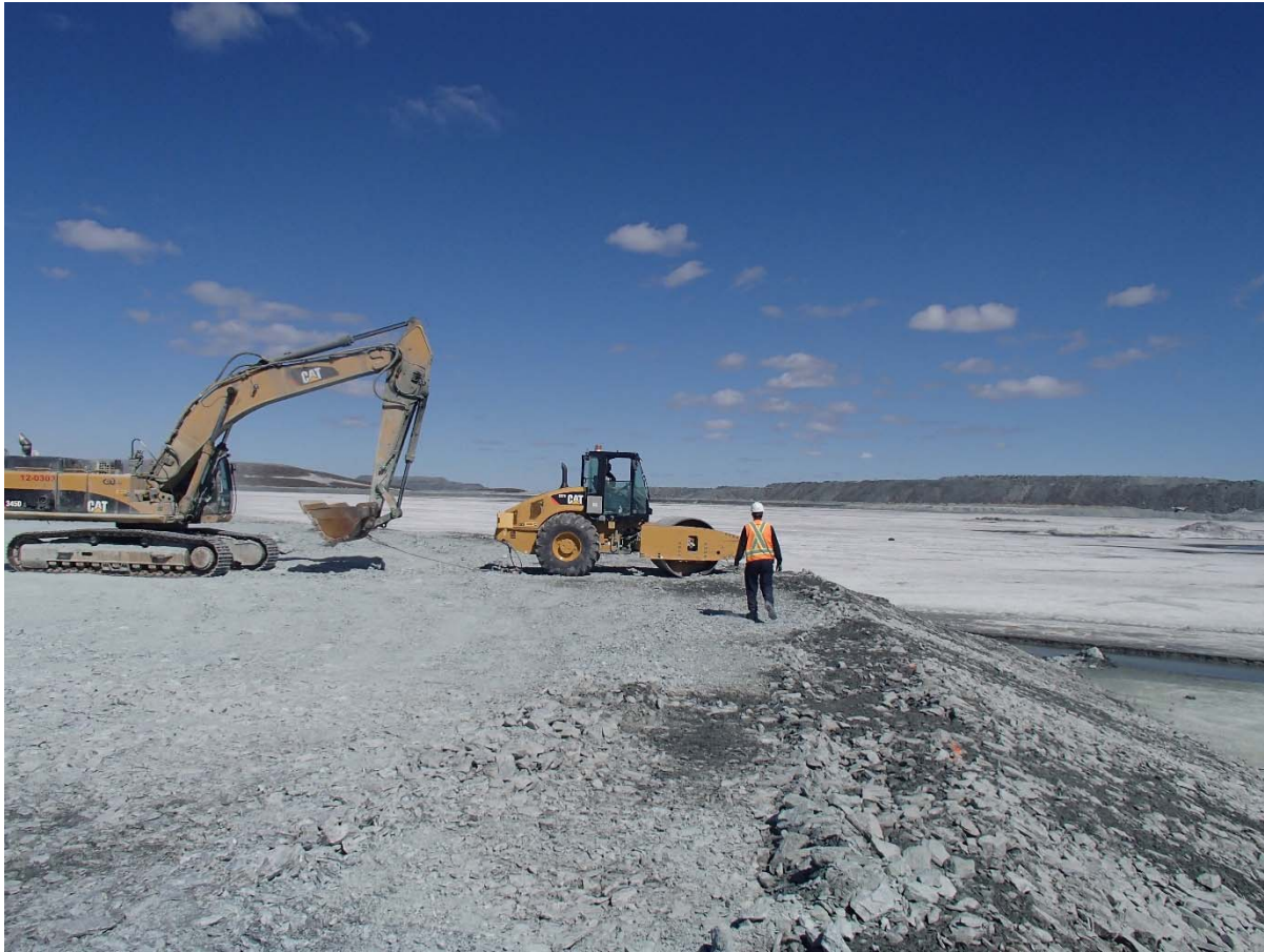
Photograph NCIS-065: From Sta. 1+140/96 m (approx.), looking NE. Compaction of the 0.5 m lift of coarse filter between El. 148 and 152 m with a 10-tonne smooth-drum compactor with vibration (4 passes) in the upstream slope from Sta. 1+270 m to 1+100 m.
