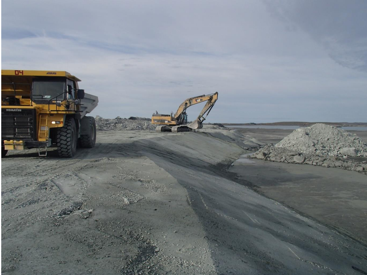
Photograph NCIS-081: From Sta2+975/-37 m (approx.), looking SE. Placement of a 0.5 m thick lift of fine filter over the coarse filter in the upstream slope from El. 150 m to 152 m with an excavator from Sta. 1+300 m to 1+210 m and from Sta. 2+940 m to 3+120 m.
