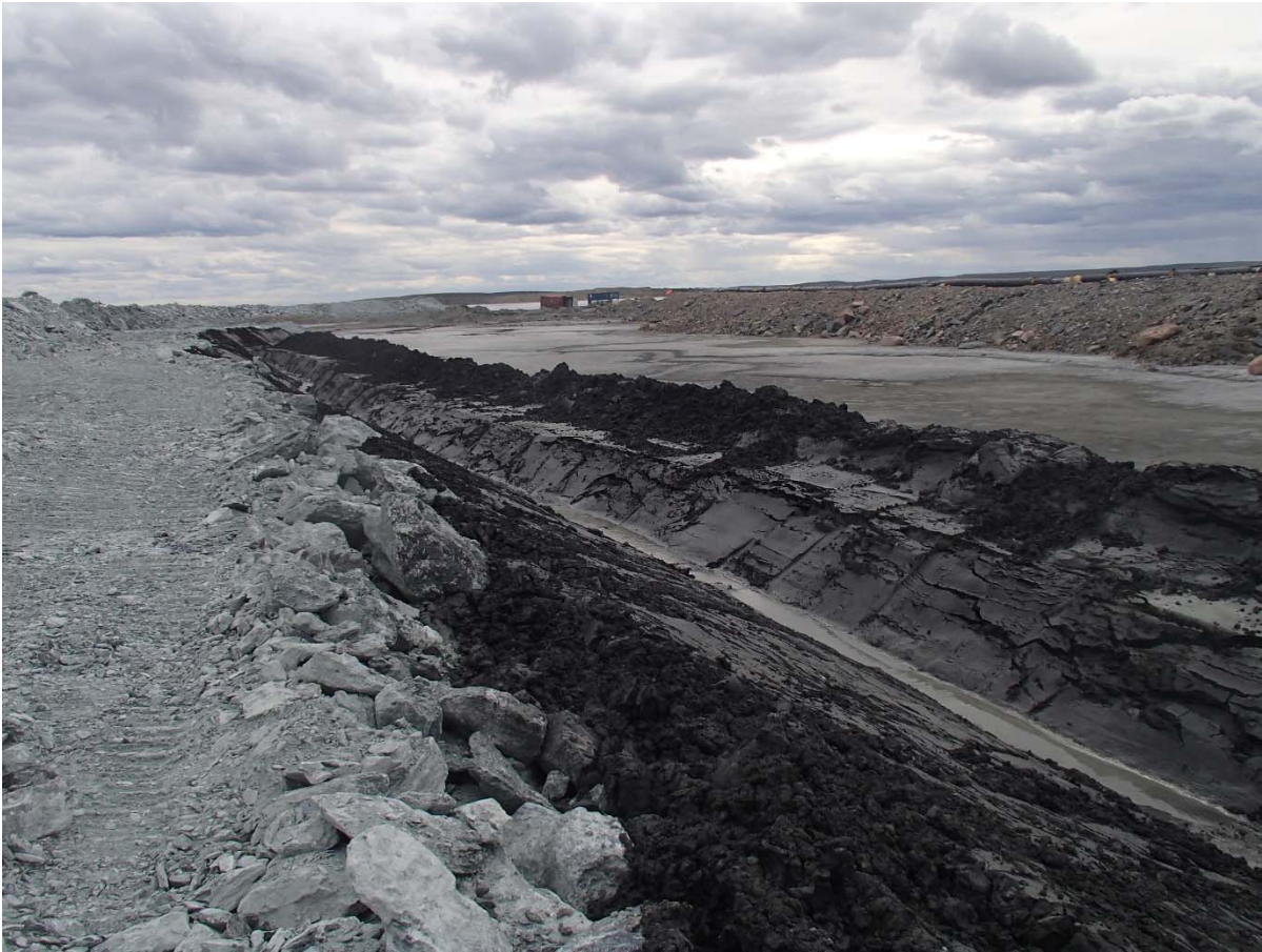
Photograph NCIS-137: From Sta. 1+380/+14 m (approx.), looking SW. Excavation of a 0.8 m (approx.) deep, 1 m wide shallow ditch in the tailings with an excavator from Sta. 1+300 m to 1+200 m.
