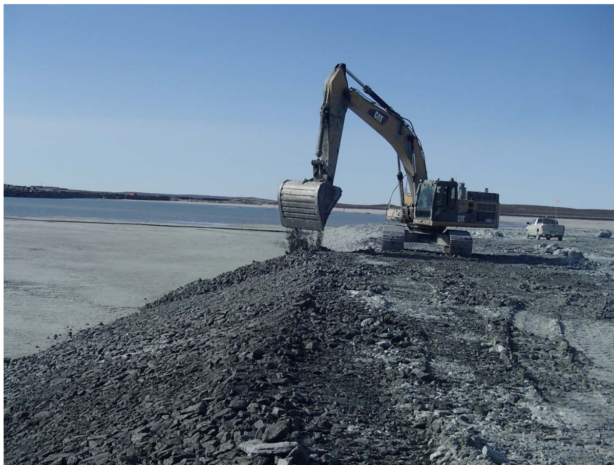
Photograph NCIS-063: From Sta. 1+200/-65 m (approx.), looking SW. Placement of a 0.5 m thick lift of coarse filter in the upstream slope from El. 148 m to 150 m with an excavator from Sta. 1+270 m to 1+100 m.
