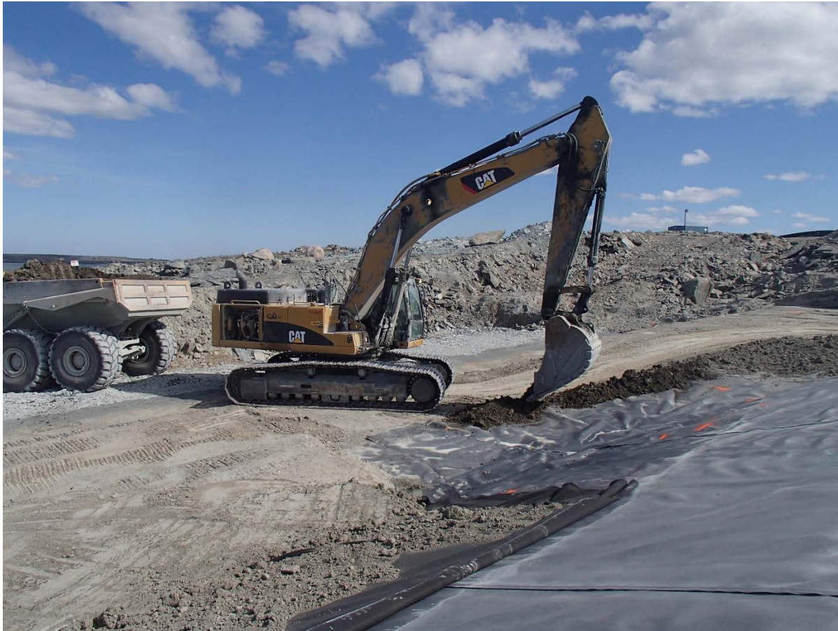
Photograph SD3-332: From Sta. 20+775/-23 m, looking SE. Placement of a first 0.5 m thick lift of compacted sieved till over the LLDPE geomembrane on the upstream toe liner tie-in with an excavator from Sta. 20+775 m to 20+800 m.
