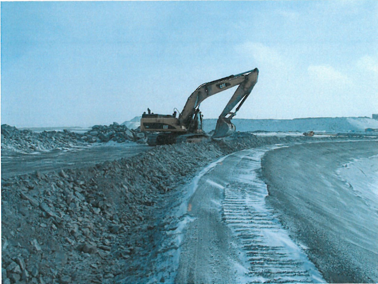
Photograph CD-1851: From Sta. 0+910/-18 m, looking S. Excavation of the LLDPE geomembrane crest anchoring trench from Sta. 40+730 m to 0+830 m.
