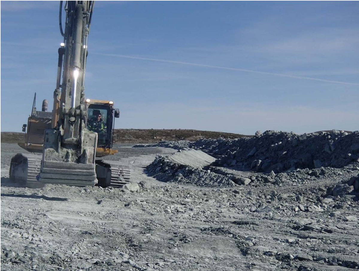
Photograph NCIS-119: From Sta. 1+430/-22 m (approx.), looking N. Excavation of a 0.8 m (approx.) deep, 1 m wide shallow ditch in the rockfill capping with an excavator from Sta. 1+455 m to 1+400 m.
