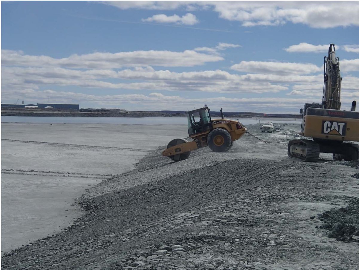
Photograph NCIS-061: From Sta. 1+365/-35 m (approx.), looking S. Compaction of the 0.5 m lift of coarse filter between El. 148 and 152 m with a 10-tonne smooth-drum compactor with vibration (4 passes) in the upstream slope from Sta. 1+340 m to 1+270 m.
