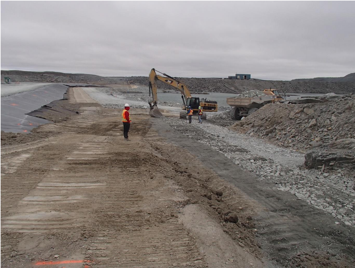
Photograph SD3-333: From Sta. 20+817/-29 m, looking N. Placement of a second 0.5 m thick lift of fine rockfill on the upstream slope of the upstream toe liner tie-in with an excavator from Sta. 20+775 m to 20+800 m.
