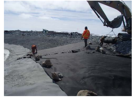
SD3-308 (2018-06-06), looking SW from Sta. 20+620/-48 m. Installation of the geotextile on the upstream slope 3H:1V between El. 143 m and 145 m from Sta. 20+620 m to 20+630 m.
