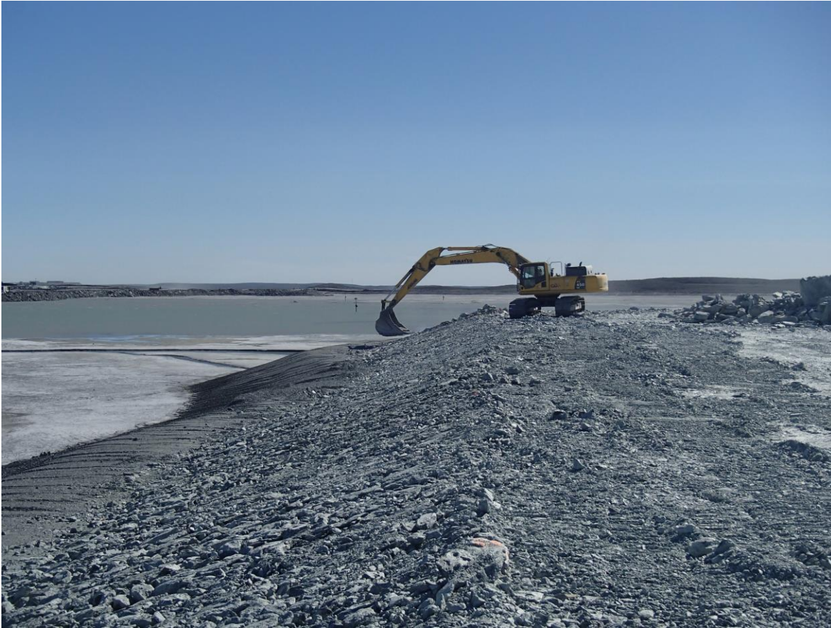
Photograph NCIS-092: From Sta 1+160/-77 m (approx.), looking S. Profiling of the upstream slope (3H:1V) from El. 150 to 152 m with an excavator from Sta. 1+185 m to 1+135 m.
