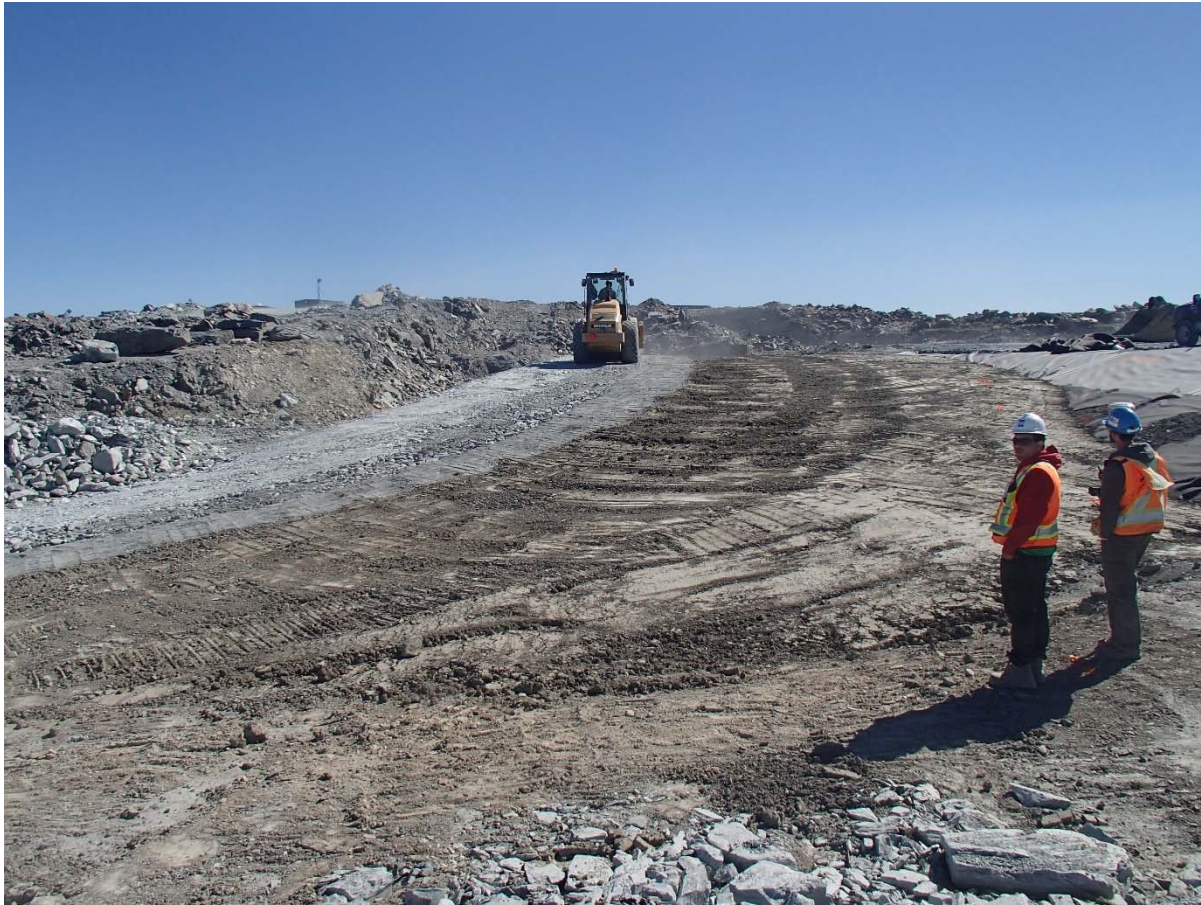
Photograph SD3-337: From Sta. 20+760/-37 m, looking S. Compaction of the fourth 0.5 m thick lifts of fine filter, coarse filter and fine rockfill on the upstream slope of the upstream toe liner tie-in with a 10-tonne smooth-drum compactor with vibrations (4 passes) from Sta. 20+770 to 20+800 m.
