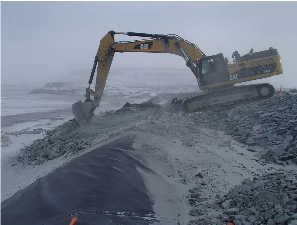
Photograph CD-1830: From Sta. 0+420/-26 m, looking N. Removal of the deposition point finger materials with an excavator at Sta. 0+390 m.
