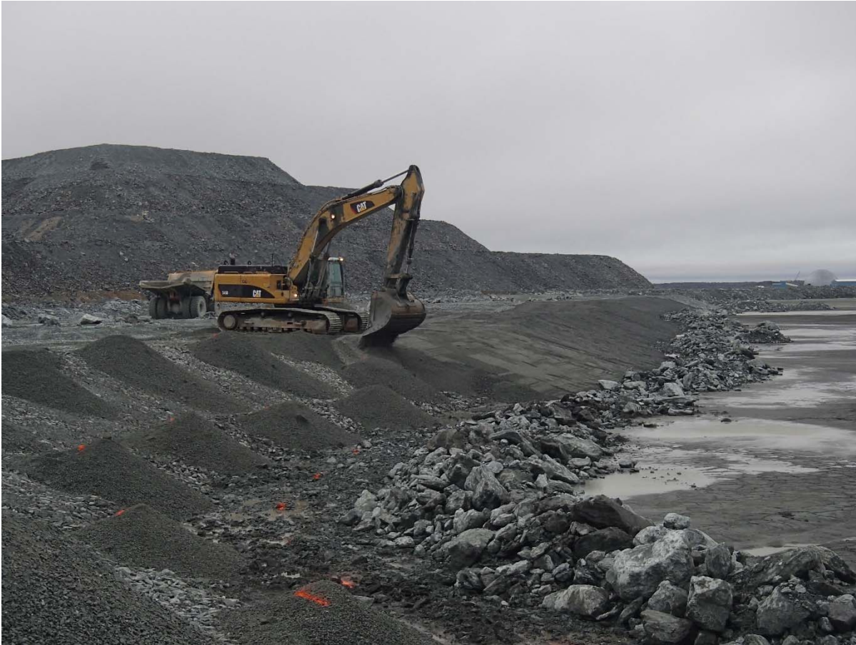
Photograph NCIS-042: From Sta. 2+210/-27 m (approx.), looking SE. Placement of a 0.5 m thick lift of fine filter over the coarse filter in the upstream slope from El. 150 m to 152 m with an excavator from Sta. 2+305 m to 2+040 m.
