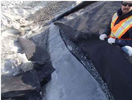
CD-1889 (2018-06-04), looking N from Sta. 0+150/-28 m. View of the underlying liner that has been cut at around Sta. 0+160 m to drain the water.
