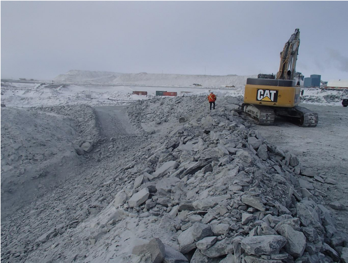
Photograph CD-1813: From Sta. 0+980/-2, looking S. Placement of intermediate volcanic (IV) rockfill on the existing downstream slope up to approx. El. 143 m, from approx. Sta. 0+980 to 40+780 m.
