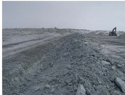
SD3-301 (2018-05-17), looking SE from Sta. 20+660/-22 m. Excavation of the LLDPE geomembrane crest anchoring trench with an excavator from Sta. 20+655 m to 20+675 m.
