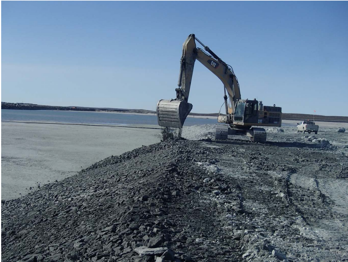
Photograph NCIS-063: From Sta. 1+200/-65 m (approx.), looking SW. Placement of a 0.5 m thick lift of coarse filter in the upstream slope from El. 148 m to 152 m with an excavator from Sta. 1+270 m to 1+100 m.
