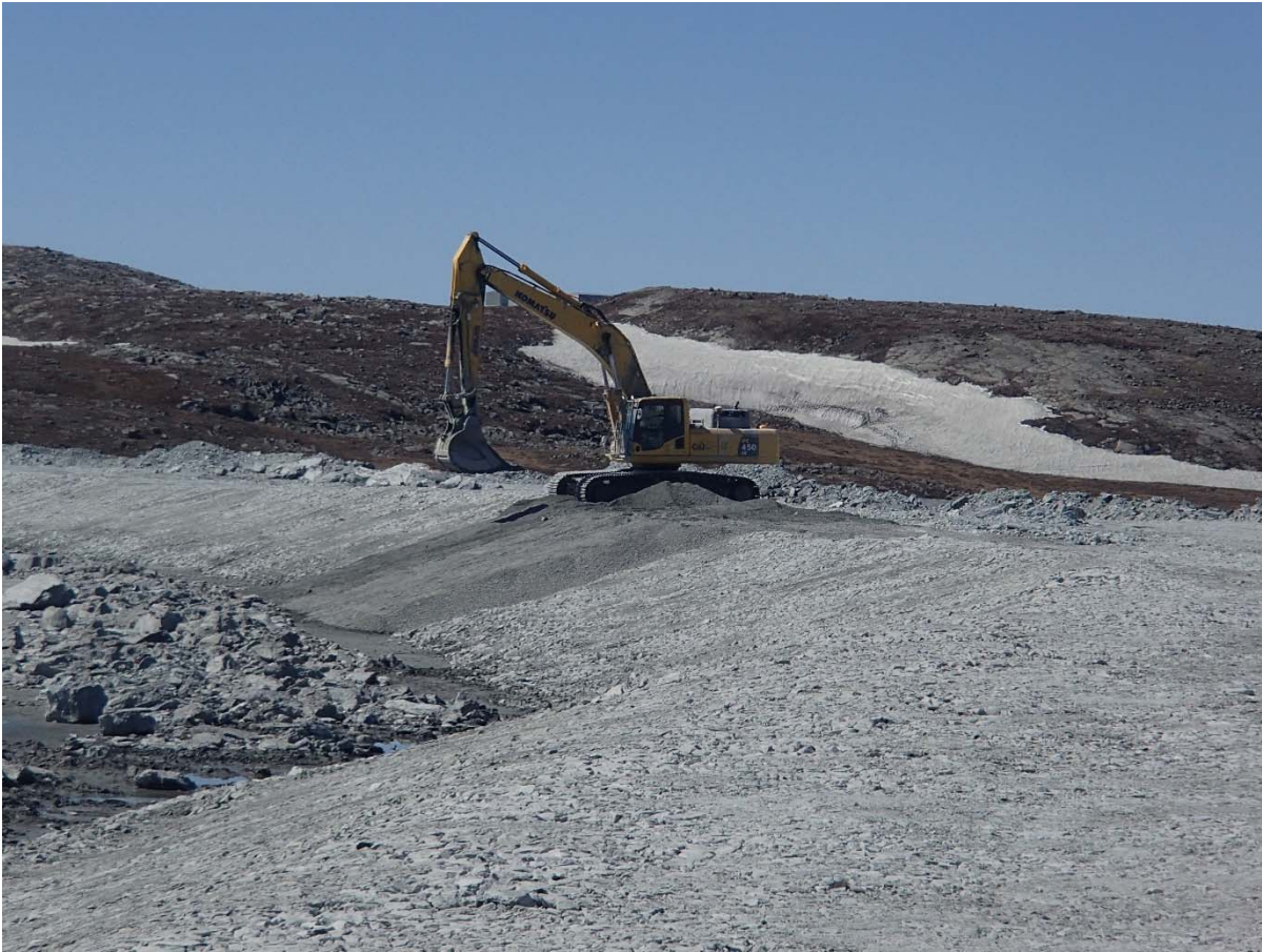
Photograph NCIS-039: From Sta. 2+200/24 m (approx.), looking W. Placement of a 0.5 m thick lift of fine filter over the coarse filter in the upstream slope from El. 150 m to 152 m with an excavator from Sta. 2+460 m to 2+475 m and from Sta. 2+065 m to 1+980 m.
