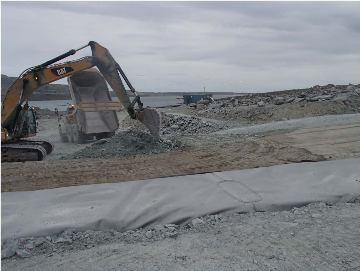
Photograph SD3-346: From Sta. 20+760/-21 m, looking E. Placement of a third 0.5 m thick lift of fine UM rockfill (0-500 mm) upstream of the low quality till (0-150mm) from El. 143 m to 143.5 m from Sta. 20+668 m to 20+777 m.
