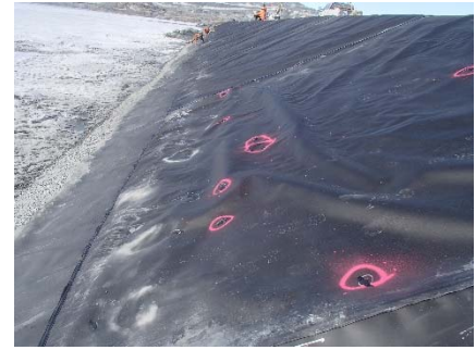
CD-1879 (2018-06-01), looking N from Sta. 0+735/-28 m. View of the repaired holes on panel 850.
