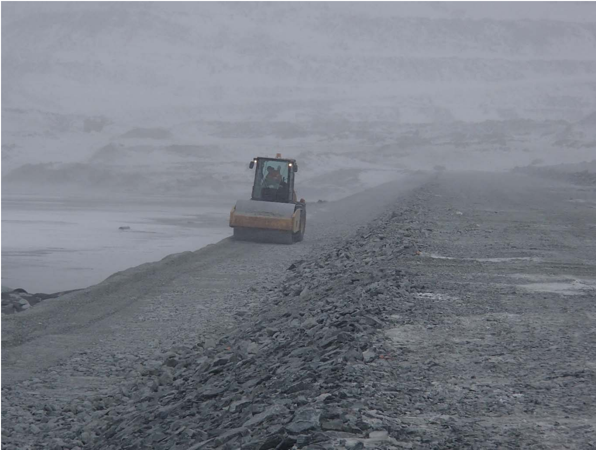
Photograph CD-1835: From Sta. 0+830/-20 m, looking N. Compaction of the first 0.5 m lift (approx.) of fine and coarse filters material at El. 143.5 m with a 10-tonne smooth-drum compactor with vibration (6 passes) from Sta. 0+490 to 0+835 m.
