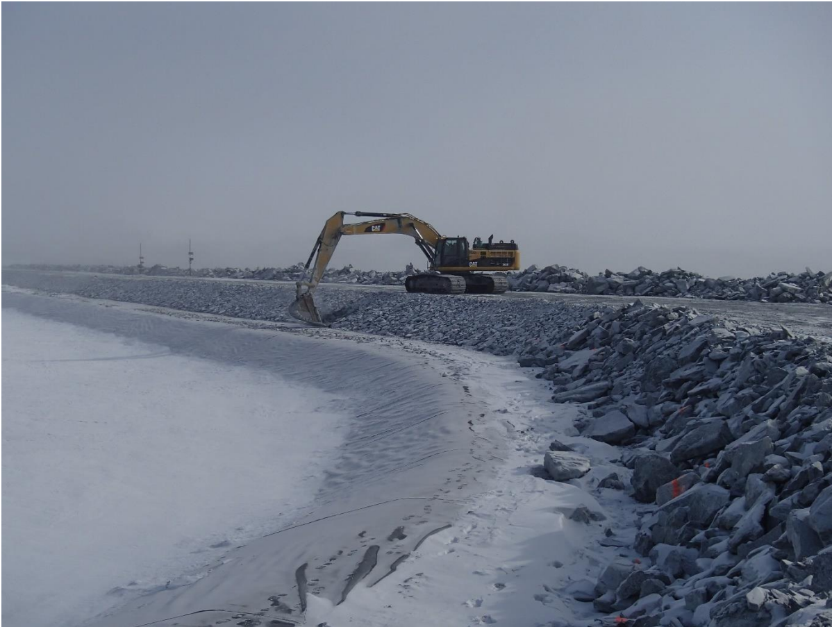
Photograph CD-1824: From Sta 40+760/-25 m, looking NE. Profiling of the upstream slope (2H:1V) from El. 143 to 145 m with an excavator between Sta. 0+830 m and 40+730 m.
