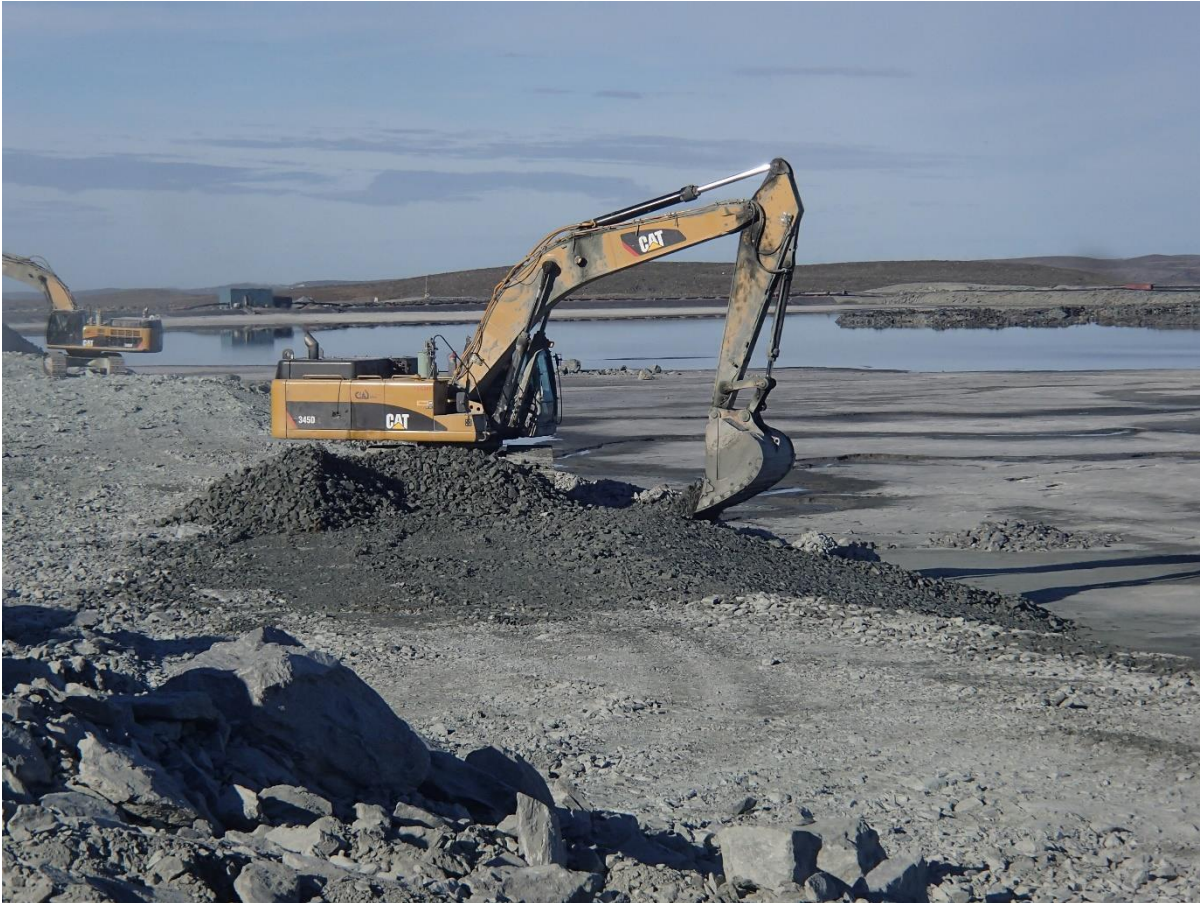
Photograph NCIS-076: From Sta. 2+940/-15 m (approx.), looking SW. Placement of a 0.5 m thick lift of coarse filter in the upstream slope from El. 150 m to 152 m with an excavator from Sta. 2+980 m to 3+160 m.
