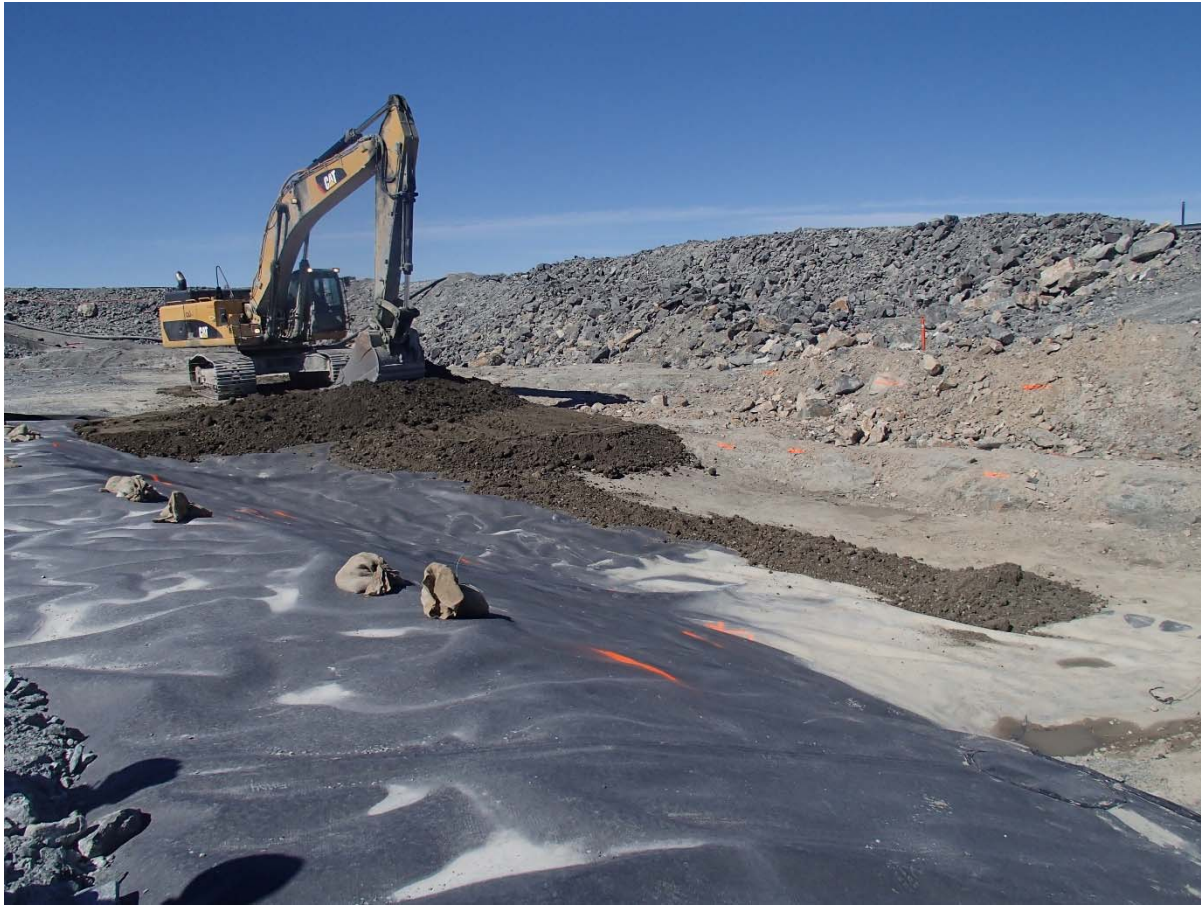
Photograph SD3-338: From Sta. 20+610/-43 m, looking NW. Placement of a first 0.5 m thick lift of compacted sieved till over the LLDPE geomembrane on the upstream toe liner tie-in with an excavator from Sta. 20+588 m to 20+599 m.
