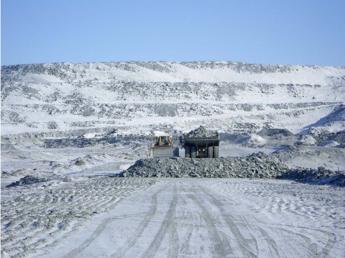
Photograph CD-1798: From Sta. 0+500/-15 m looking N. Placement a 2 m thick (approx.) lift of volcanic rockfill from El. 143 m to El. 145 m from 0+340 to 0+435 m (o.s. -28 to -18 m).
