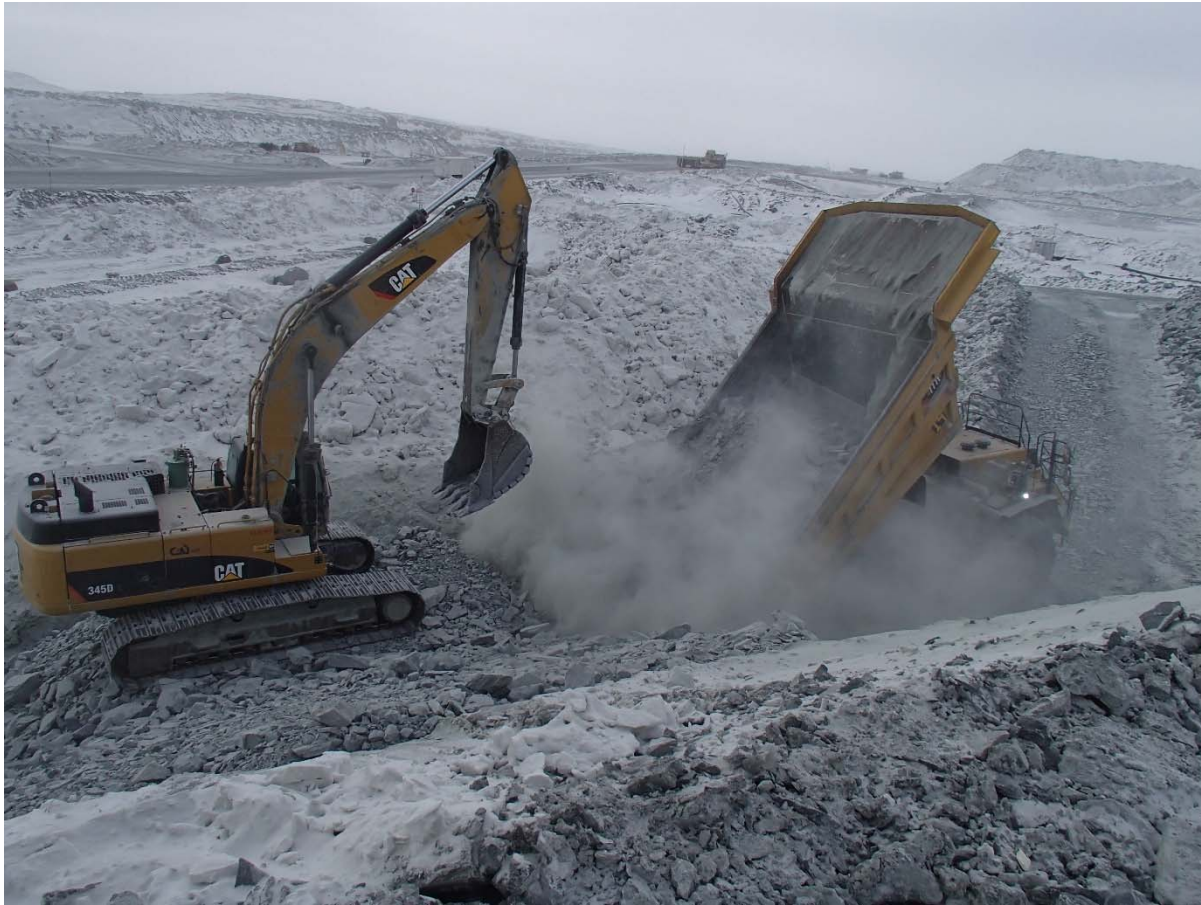
Photograph CD-1811: From Sta. 0+985/-11 m looking SE. Placement the second, third, fourth and fifth 1 m thick (approx.) lifts of intermediate volcanic (IV) rockfill from approx. Sta. 0+985 to 40+780 m (o.s. -8 to 8 m) with the excavator.
