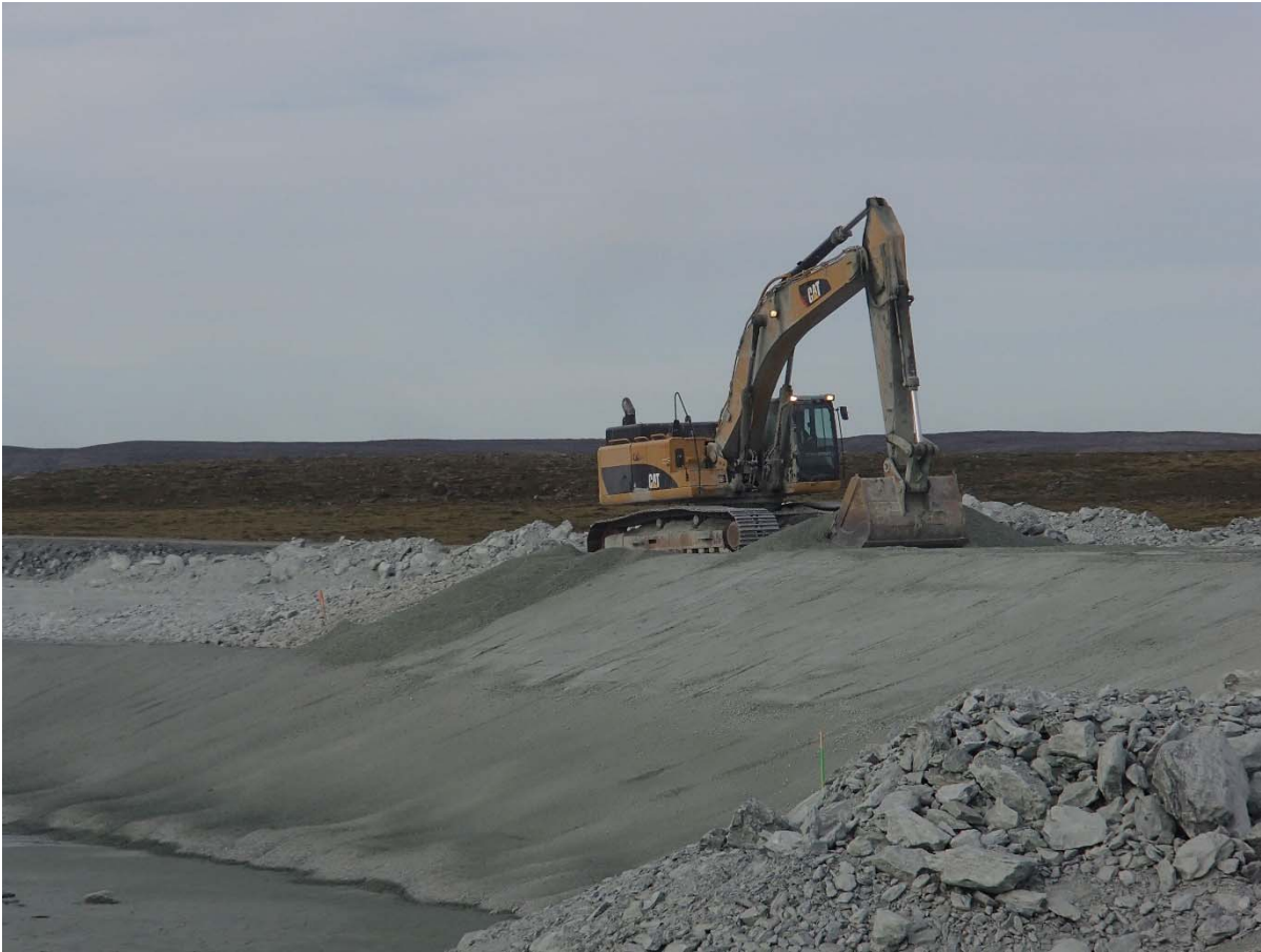
Photograph NCIS-136: From Sta. 1+800/-33 m (approx.), looking SW. Placement of a 0.5 m thick lift of fine filter in the upstream slope from El. 152 m to 154 m with an excavator from Sta. 1+700 m to 1+660 m.
