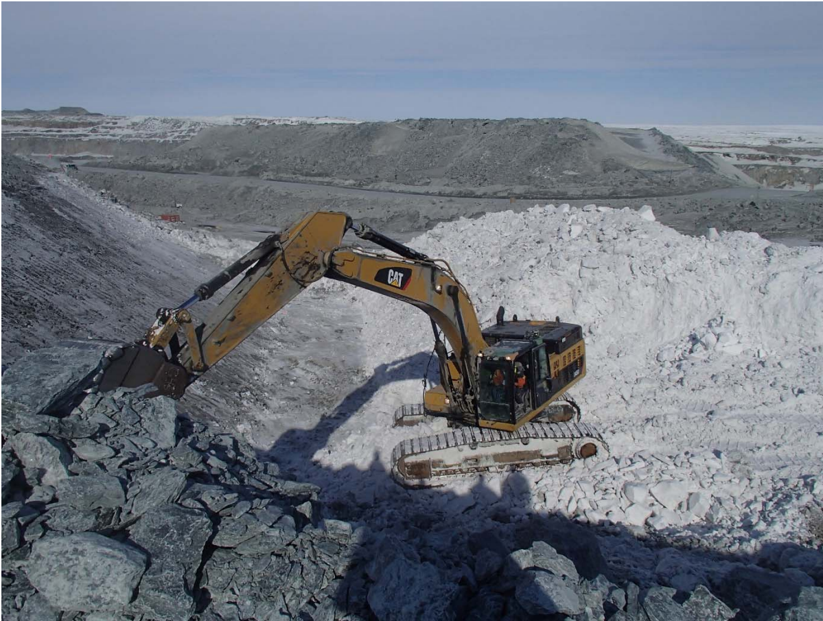
Photograph CD-1803: From Sta. 40+750/27 m looking NE. Removal of snow to expose the foundation bedrock with an excavator between approx. Sta. 40+780 and 40+800 m (o.s. 7 to 10 m).
