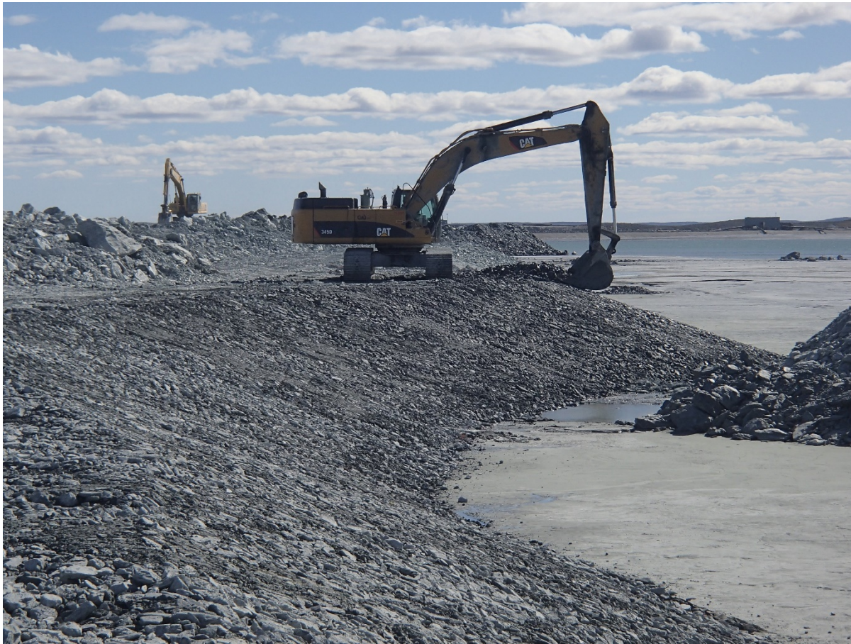
Photograph NCIS-075: From Sta. 2+860/-36 m (approx.), looking S. Placement of a 0.5 m thick lift of coarse filter in the upstream slope from El. 150 m to 152 m with an excavator from Sta. 2+815 m to 2+980 m.
