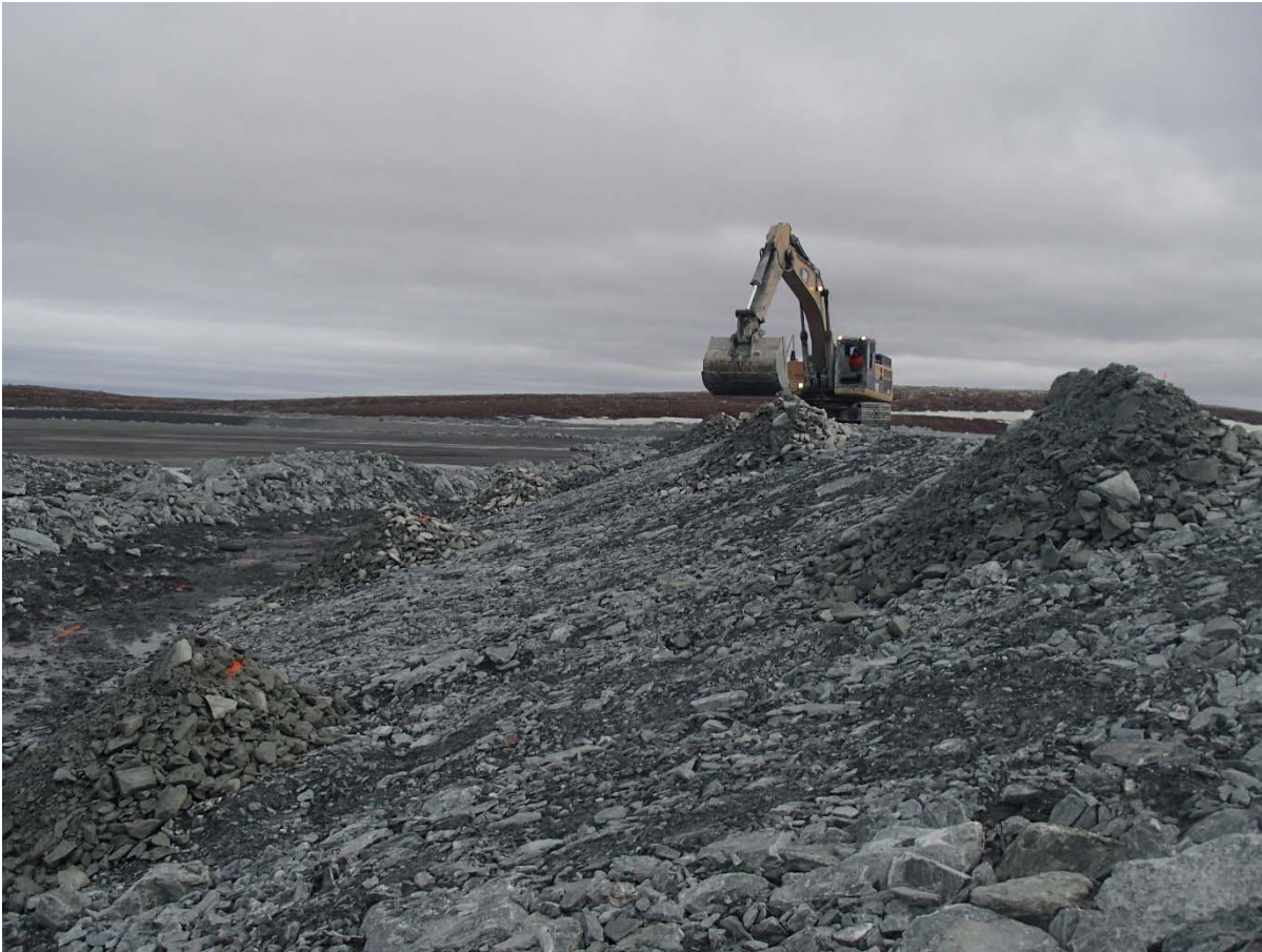
Photograph NCIS-047: From Sta. 2+580/-35 m (approx.), looking N. Placement of a 0.5 m thick lift of coarse filter in the upstream slope from El. 150 m to 152 m with an excavator from Sta. 2+560 m to 2+640 m.
