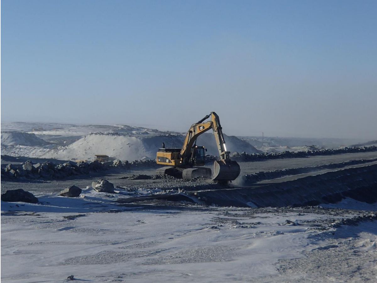
Photograph CD-1844: From Sta 0+080/-49 m, looking SW. Placement of a fourth 0.5 m thick lift of coarse filter from El. 144.5 m to 145 m with an excavator from Sta. 0+170 m to 40+730 m.
