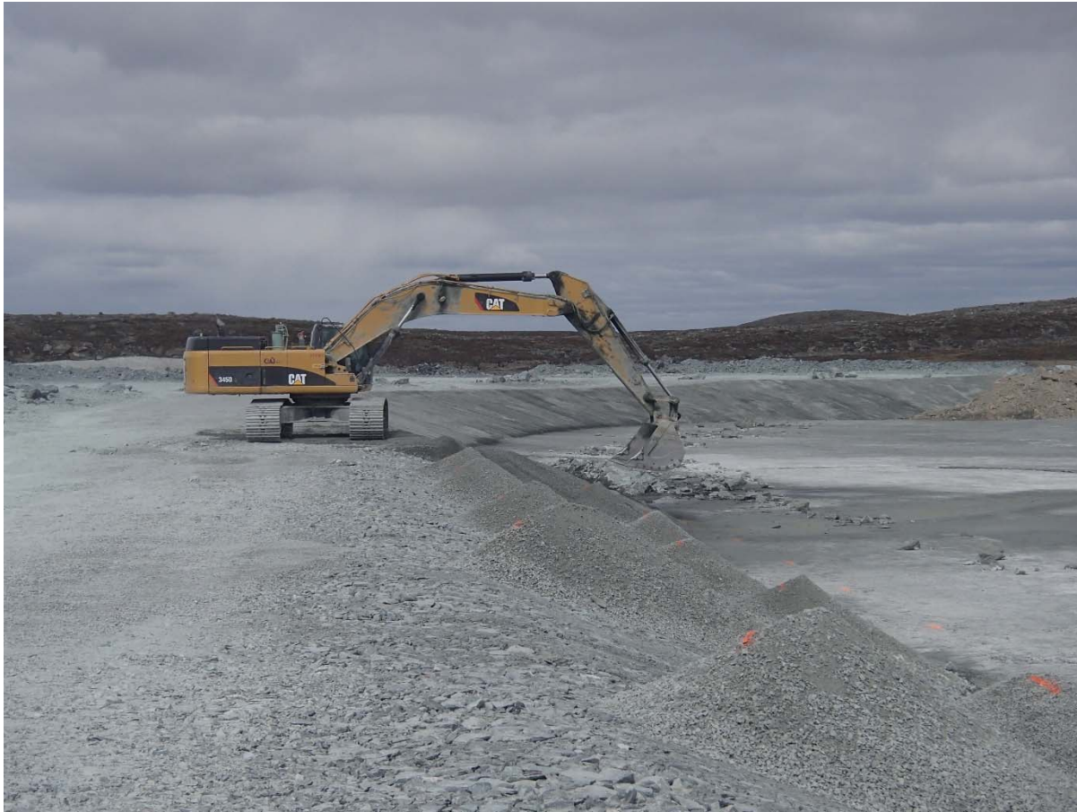
Photograph NCIS-062: From Sta. 1+525/-33 m (approx.), looking N. Placement of a 0.5 m thick lift of fine filter over the coarse filter in the upstream slope from El. 150 m to 152 m with an excavator from Sta. 1+330 m to 1+260 m and from Sta. 1+595 m to 1+550 m.
