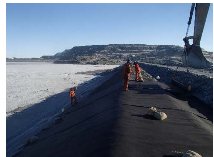
CD-1885 (2018-06-03), looking N from Sta. 0+460/-26 m. Installation of the geotextile on the upstream slope 2H:1V between El. 143 m and 145 m from Sta. 0+480 m to 0+320 m. compactor with vibration (4 passes) from Sta. 0+610 to 0+480 m.
