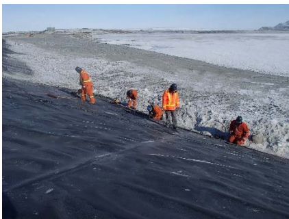
CD-1865 (2018-05-25), looking NW from Sta. 40+740/-35 m. Repairs on the extrusion fillet seam at the bottom of the LLDPE liner panels between Sta. 40+680 m and 0+950 m, on panels 802 to 807, and 811 to 813.
