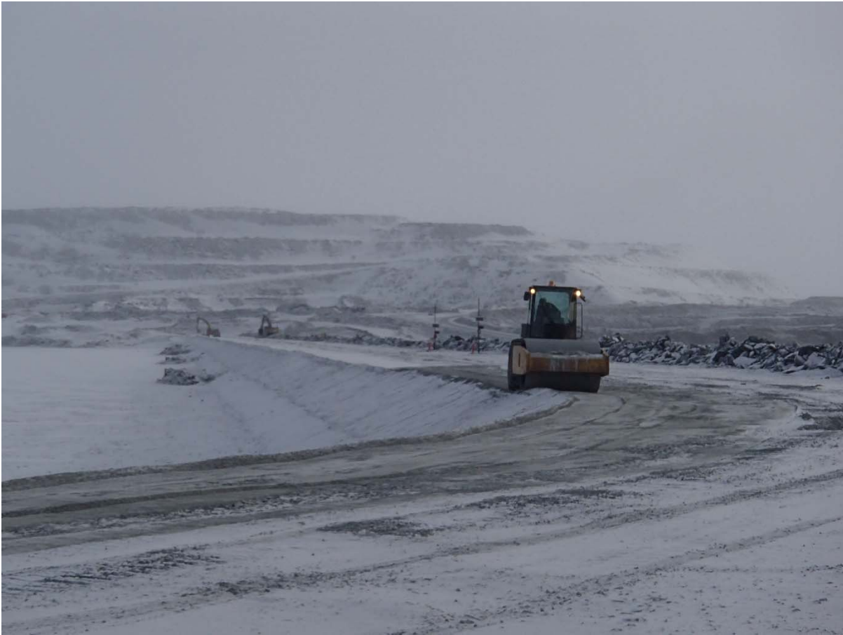
Photograph CD-1848: From Sta. 40+780/-15m, looking N. Compaction of the fourth 0.5 m lift (approx.) of fine and coarse filters material at El. 145 m with a 10-tonne smooth-drum compactor with vibration (4 passes) from Sta. 0+930 m to 40+730 m.
