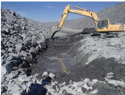
NCIS-115 (2018-07-24), looking NE from Sta. 3+040/-33 m (approx.). Excavation of a 1 m (approx.) sump in the tailings with an excavator from Sta. 3+010 m to 3+030 m (o.s. +27 to +30 m).
