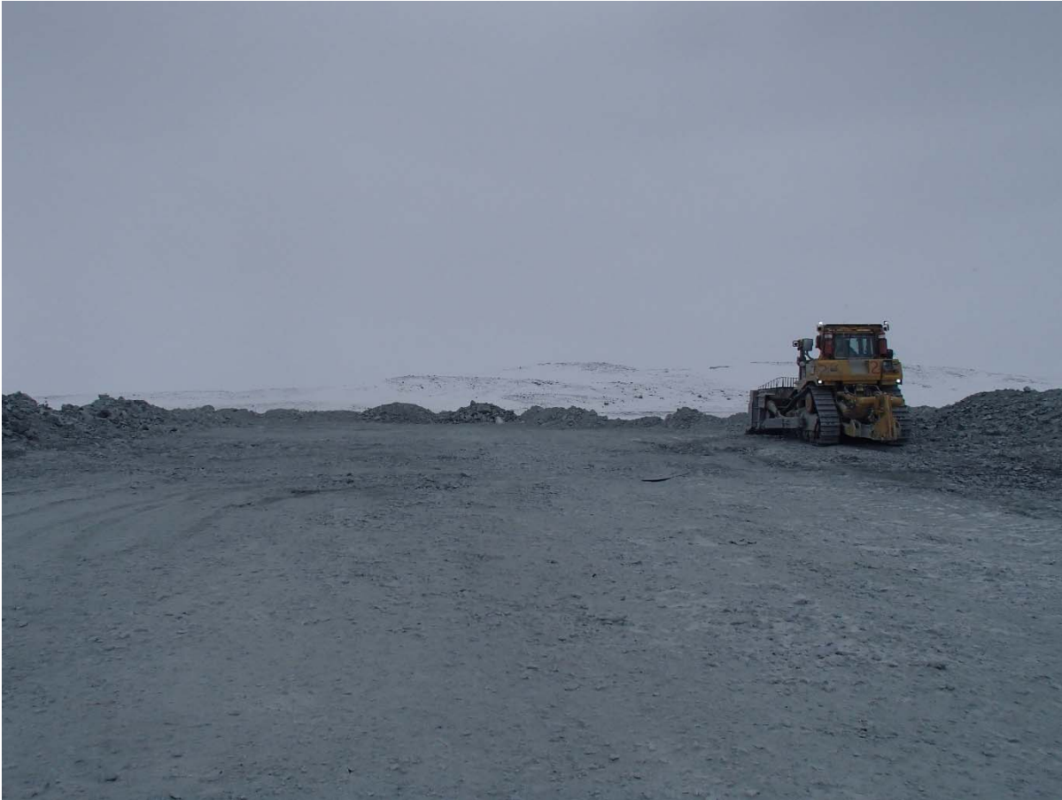
Photograph NCIS-009: Placement a 2 m thick (approx.) lift of UM rockfill from El. 150 m to El. 152 m (approx.) with a dozer from Sta. 1+880 m to 1+825 m (o.s. unavailable).
