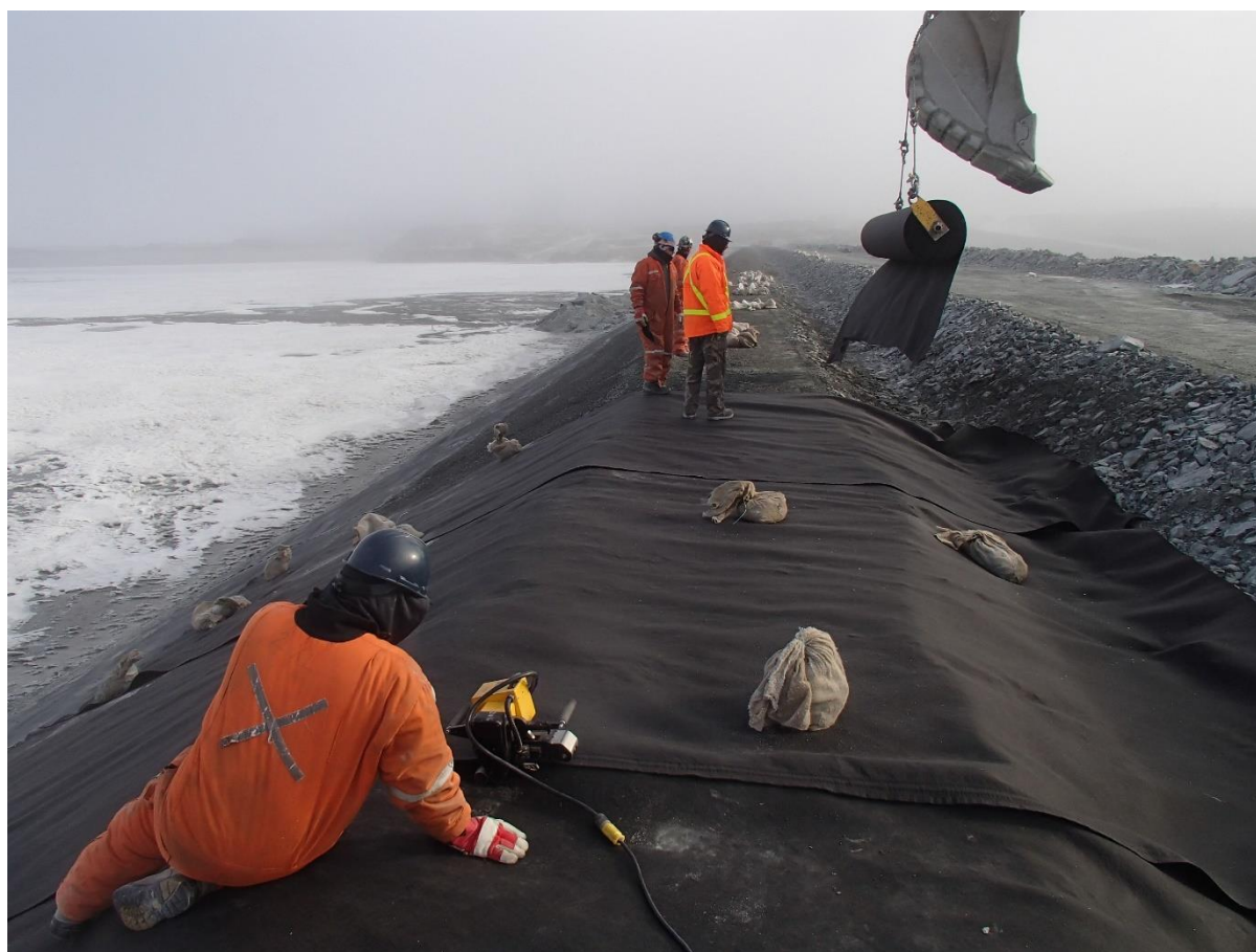
Photograph CD-1880: From Sta. 0+600/-25 m, looking N. Installation of the geotextile on the upstream slope 2H:1V between El. 143 m and 145 m from Sta. 0+610 m to 0+480 m.
