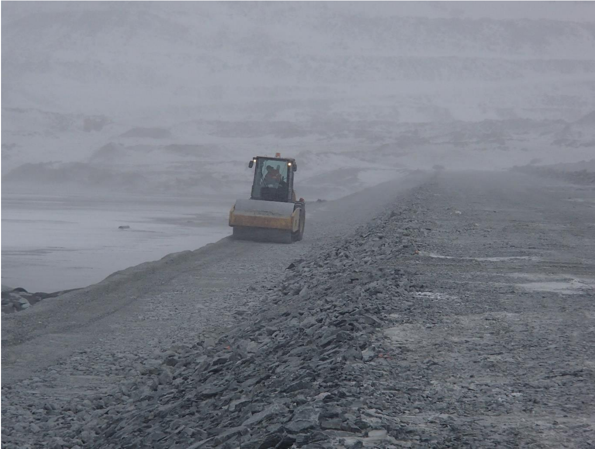
Photograph CD-1835: From Sta 0+830/-20m, looking N. Compaction of the first 0.5 m lift (approx.) of fine and coarse filters material at El. 143.5 m with a 10-tonne smooth-drum compactor with vibration (6 passes) from Sta 0+490 to 0+835 m.
