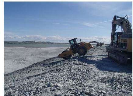
NCIS-099 (2018-07-19), looking SE from Sta. 1+180/-76 m (approx.). Compaction of the 0.5 m lift (approx.) of coarse filter between El. 150 m and 152 m with a 10-tonne smooth-drum compactor with vibration (4 passes) in the upstream slope from Sta. 1+200 m to 1+170 m.
