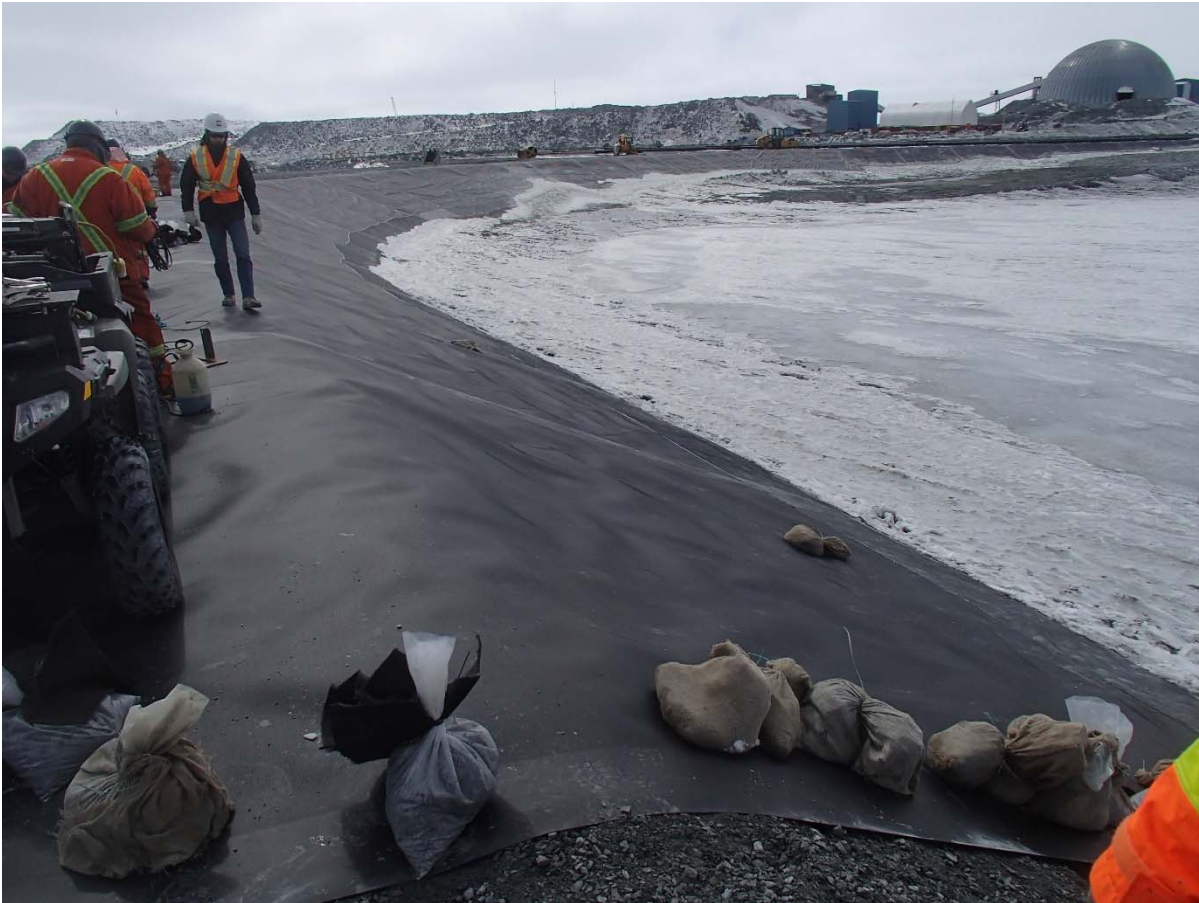
Photograph CD-1870: From Sta. 0+900/-26 m, looking S. Installation of the LLDPE liner on the upstream slope 2H:1V between El. 143 m and 145 m from Sta. 0+935 m to 0+900 m (panel numbers 820 to 823).
