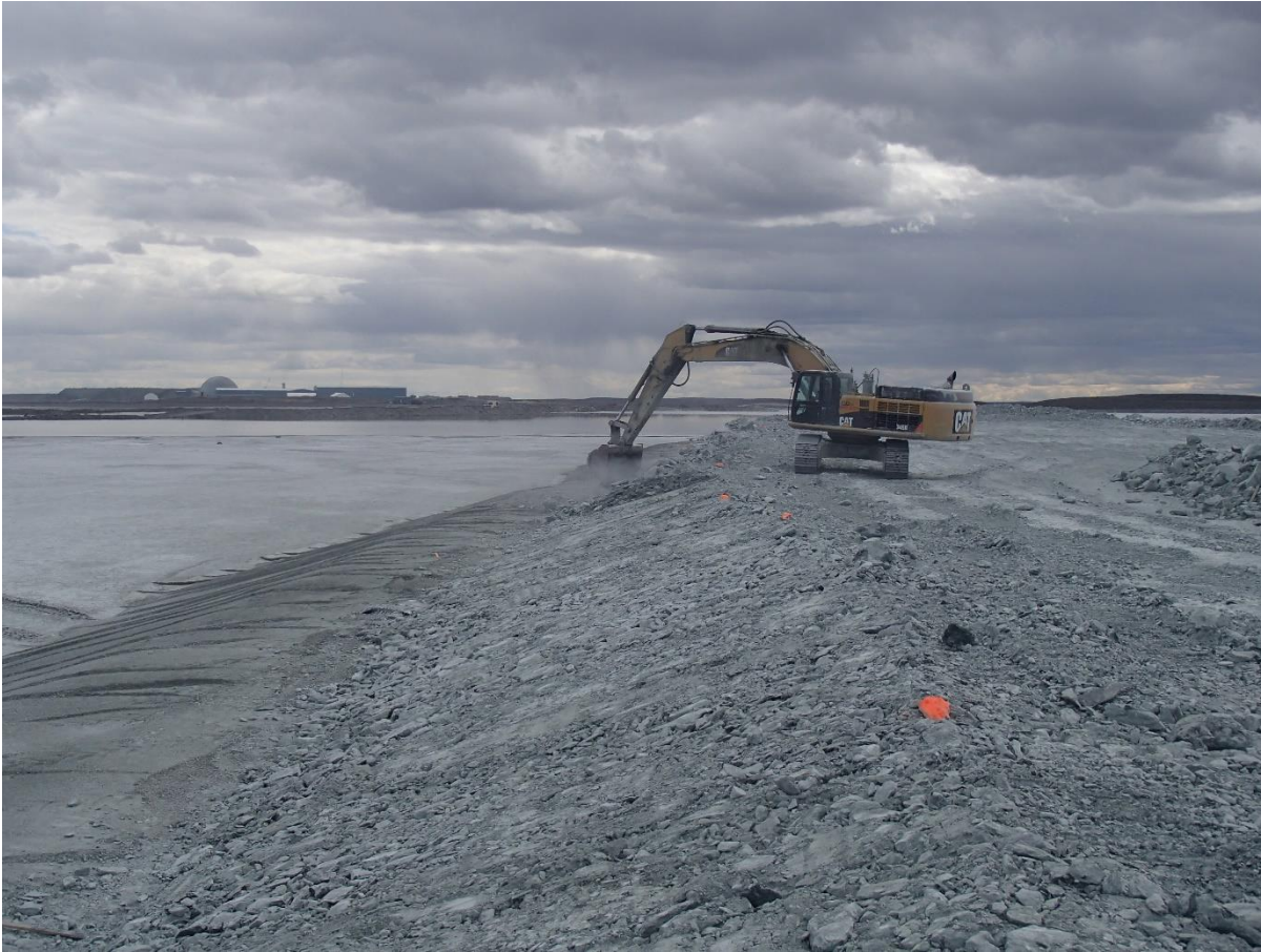
Photograph NCIS-077: From Sta. 1+310/-32 m (approx.), looking S. Profiling of the upstream slope (3H:1V) from El. 150 to 152 m with an excavator from Sta. 1+300 m to 1+175 m and from 3+070 m to 3+160 m.
