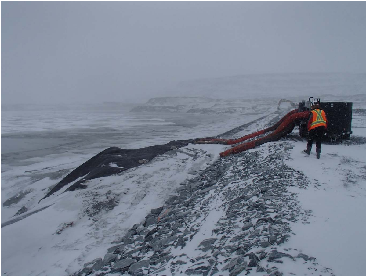
Photograph CD-1828: From Sta 0+410/-22 m, looking N. Defrosting of the deposition finger materials with two Frost Fighters at Sta. 0+390 m.
