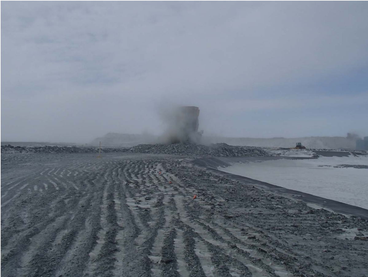
Photograph CD-1815: From Sta. 0+920/-25, looking S. Placement of a 2 m thick (approx.) lift of intermediate volcanic (IV) rockfill from El. 143 m to El. 145 m from approx. Sta. 40+740 to 0+980 m (o.s. -28 to -11 m).
