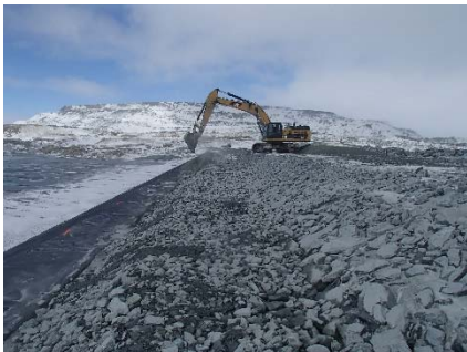
CD-1829 (2018-05-06), looking N from Sta. 0+340/-24 m. Placement of a 0.5 m thick lift of coarse filter from El. 143 m to 143.5 m with an excavator from Sta. 0+170 m to 0+460 m and placement of a 0.5 m thick lift of fine filter from Sta. 0+170 m to 0+380 m.
