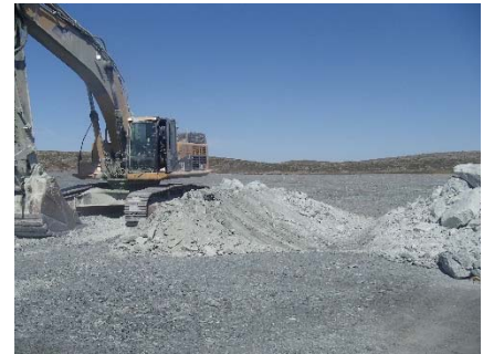
NCIS-114 (2018-07-24), looking N from Sta. 1+700/-34 m (approx.). Excavation of a 0.8 m (approx.) deep, 1 m wide shallow ditch in the rockfill capping with an excavator from Sta. 1+500 m to 1+650 m.
