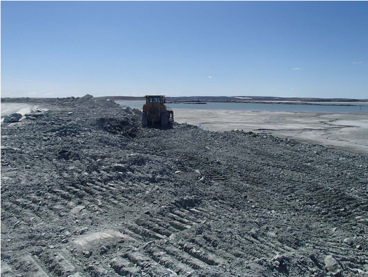
Photograph NCIS-057: From Sta. 3+010/-15 m (approx.), looking SW. Removing of UM rockfill material from the capping with a dozer to level the surface to El. 152 m from Sta. 2+980 m to 3+050 m (offset -30 to -20 m).
