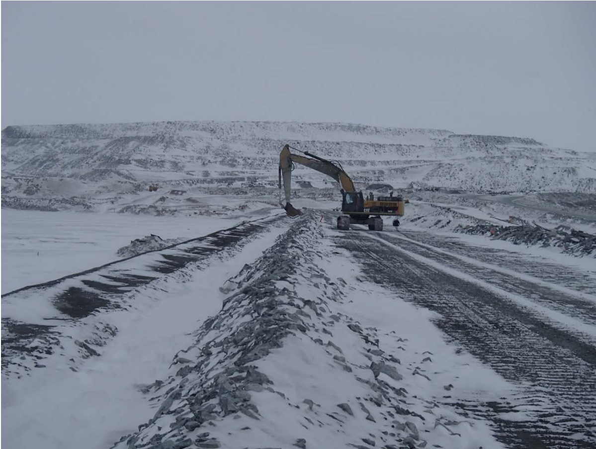
Photograph CD-1857: From Sta. 0+700/-20 m, looking N. Snow removal in the anchoring trench with an excavator between Sta. 0+170 m and 40+780 m.
