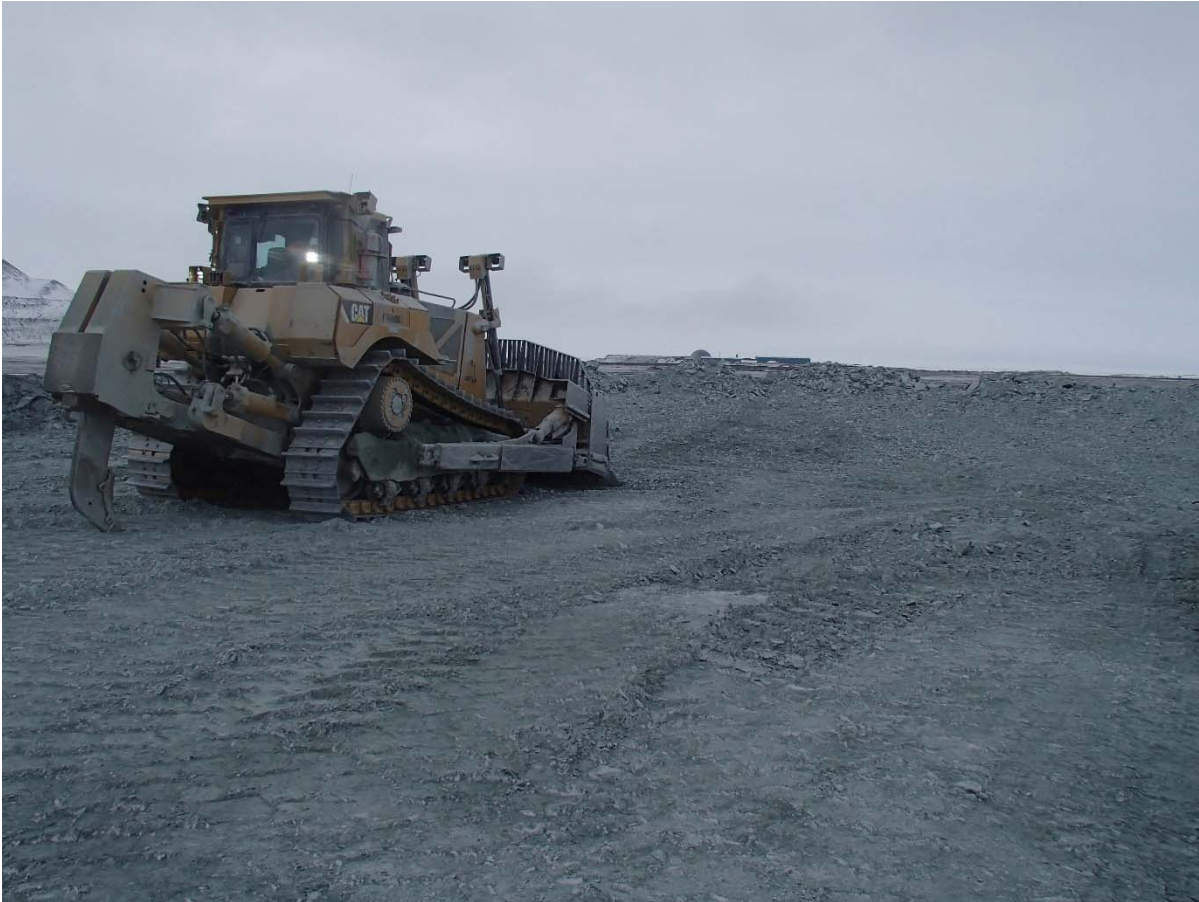
Photograph NCIS-020: From Sta. 1+570 m (approx.), looking S. Placement a 2 m thick (approx.) lift of UM rockfill from El. 150 m to El. 152 m (approx.) with a dozer from Sta. 1+564 m to 1+535 m (o.s. unavailable).
