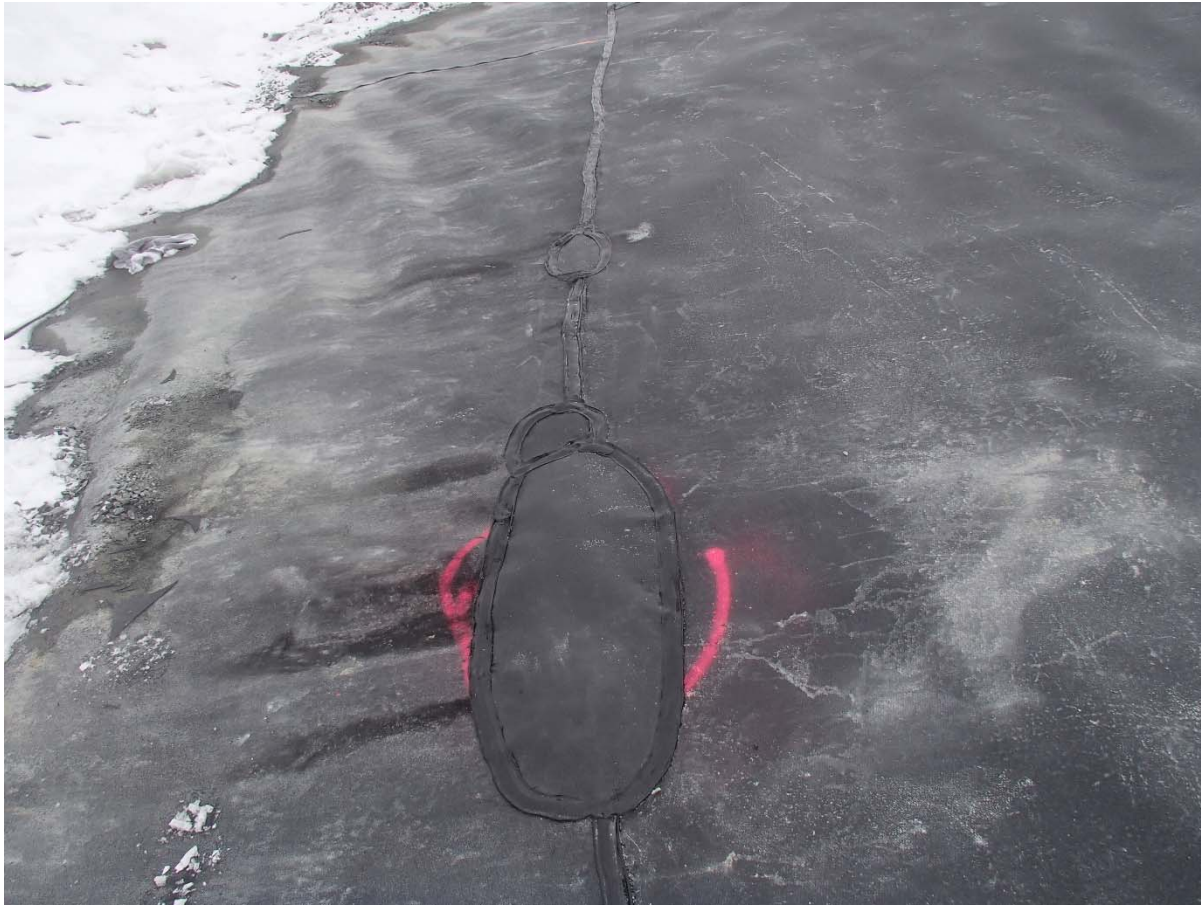
Photograph CD-1876: From Sta. 0+820/-26 m, looking N. View of repair patches on the extrusion weld at the bottom of panel 838.
