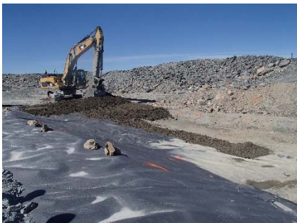
SD3-338 (2018-07-14), looking NW from Sta. 20+610/-43 m. Placement of a first 0.5 m thick lift of compacted sieved till over the LLDPE geomembrane on the upstream toe liner tie-in with an excavator from Sta. 20+588 m to 20+599 m.
