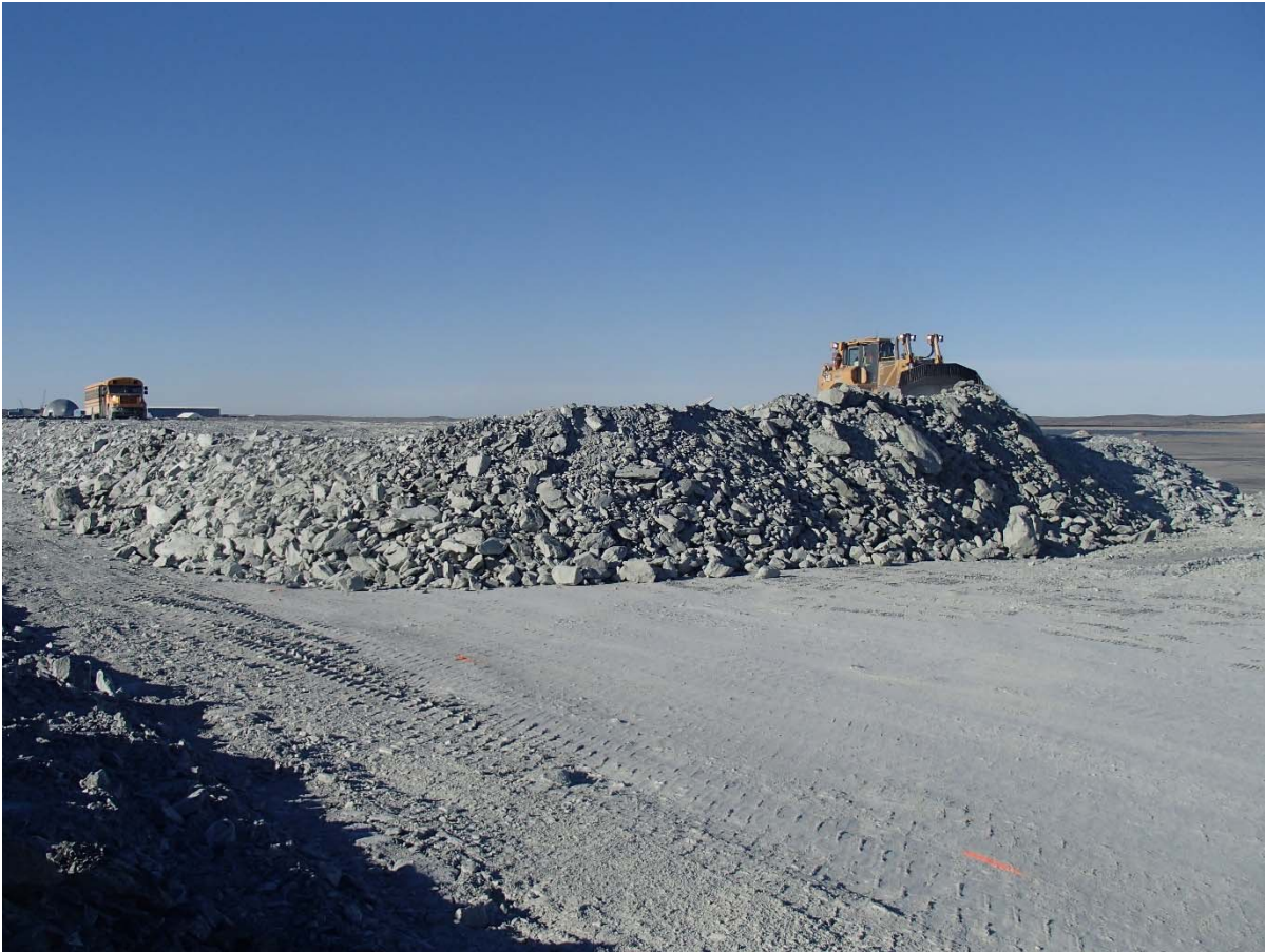
Photograph NCIS-091: From Sta 2+330/+13 m (approx.), looking S. Placement of a 2 m thick (approx.) lift of UM rockfill from El. 152 m to El. 154 m (approx.) with a dozer from Sta. 2+370 m to 2+290 m (+9 m to -22 m). The material is of good quality and is well graded.
