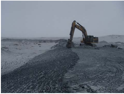
NCIS-019 (2018-05-26), looking SW from Sta. 2+100 m. Profiling of the upstream slope (3H:1V) from El. 150 to 152 m with an excavator from Sta. 1+860 m to 1+678 m. The portion between Sta. 1+900 m and 1+800 m, where the structure is built on the natural ground, was not profiled.
