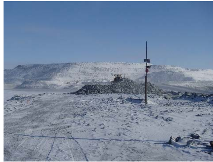
CD-1809 (2018-04-29), looking N from Sta. 0+870/-16 m. Placement a 2 m thick (approx.) lift of intermediate volcanic (IV) rockfill from El. 143 m to El. 145 m from approx. Sta. 0+760 to 0+835 m (o.s. -28 to 3 m).
