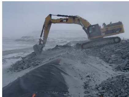
CD-1830 (2018-05-07), looking N from Sta. 0+420/-26 m. Removal of the deposition finger materials with an excavator at Sta. 0+390 m.
