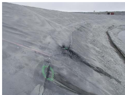
CD-1893 (2018-06-06), looking SW from Sta. 0+950/-27 m. View of repair patches on the extrusion weld at the bottom of the panels 803, 807, 808, 810, 814, 815, 816 and 818.
