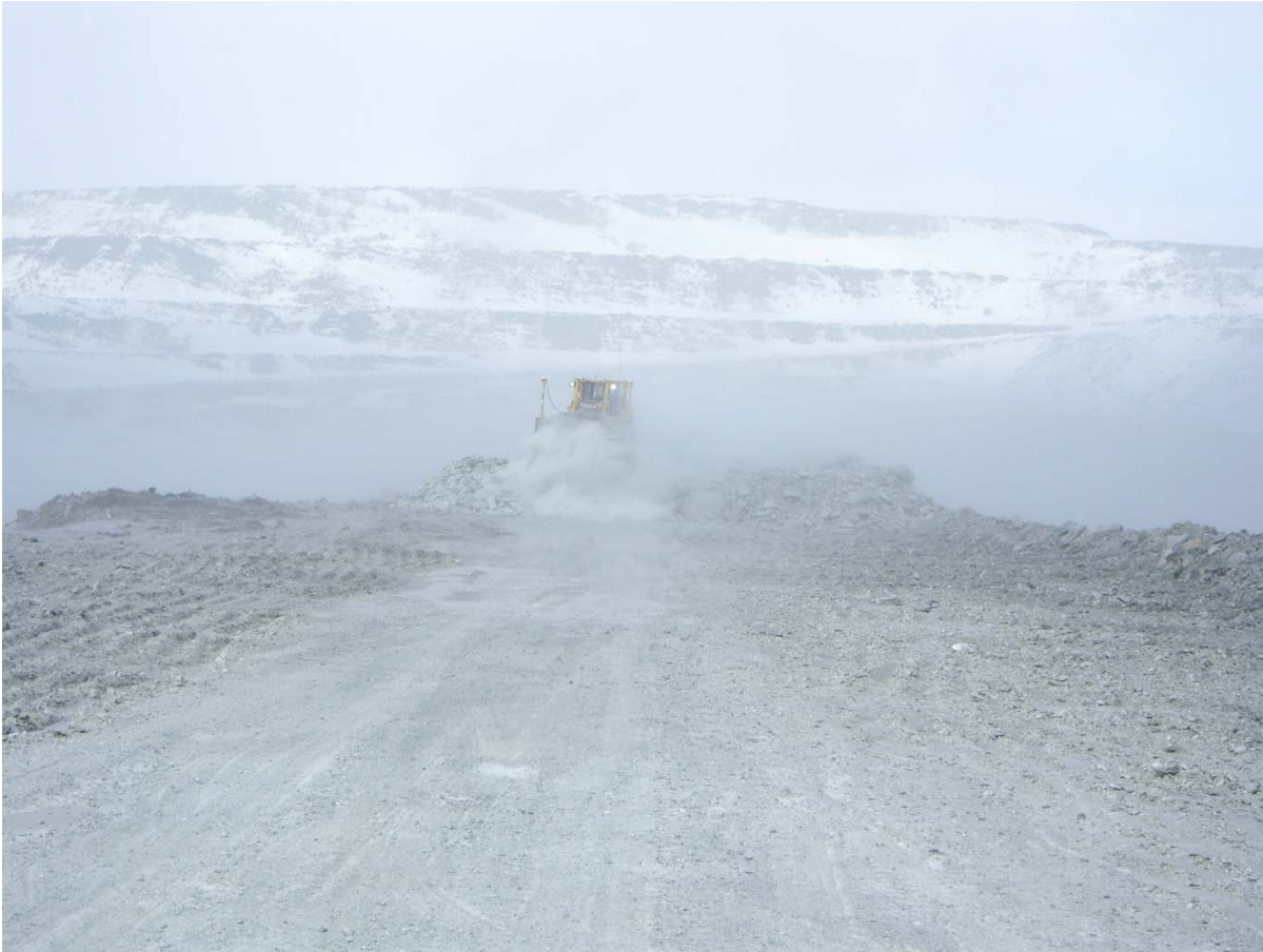
Photograph CD-1800: From Sta. 0+500/-14 m looking N. Placement a 2 m thick (approx.) lift of intermediate volcanic (IV) rockfill from El. 143 m to El. 145 m from 0+435 to 0+535m (o.s. -28 to -18 m).
