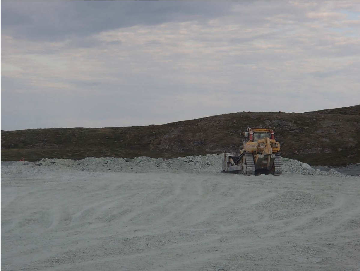
Photograph NCIS-122: From Sta. 1+960/-6 m (approx.), looking W. Placement of a 2 m thick (approx.) lift of UM rockfill from El. 152 m to El. 154 m (approx.) with a dozer from Sta. 1+830 m to 1+860 m (+8 m to -23 m).
