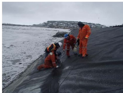
CD-1875 (2018-05-30), looking N from Sta. 0+835/-26 m. View of a vacuum box testing.
