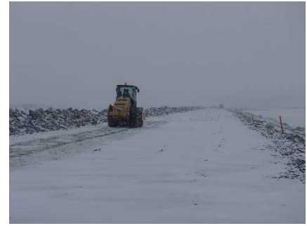
CD-1807 (2018-04-28), looking S from Sta. 0+200/-15 m. Compaction of the 2 m lift (approx.) of IV rockfill with a 10-tonne smooth-drum compactor with vibration (6 passes) from Sta. 0+150 to 0+280 m (o.s. -21 to 11 m).
