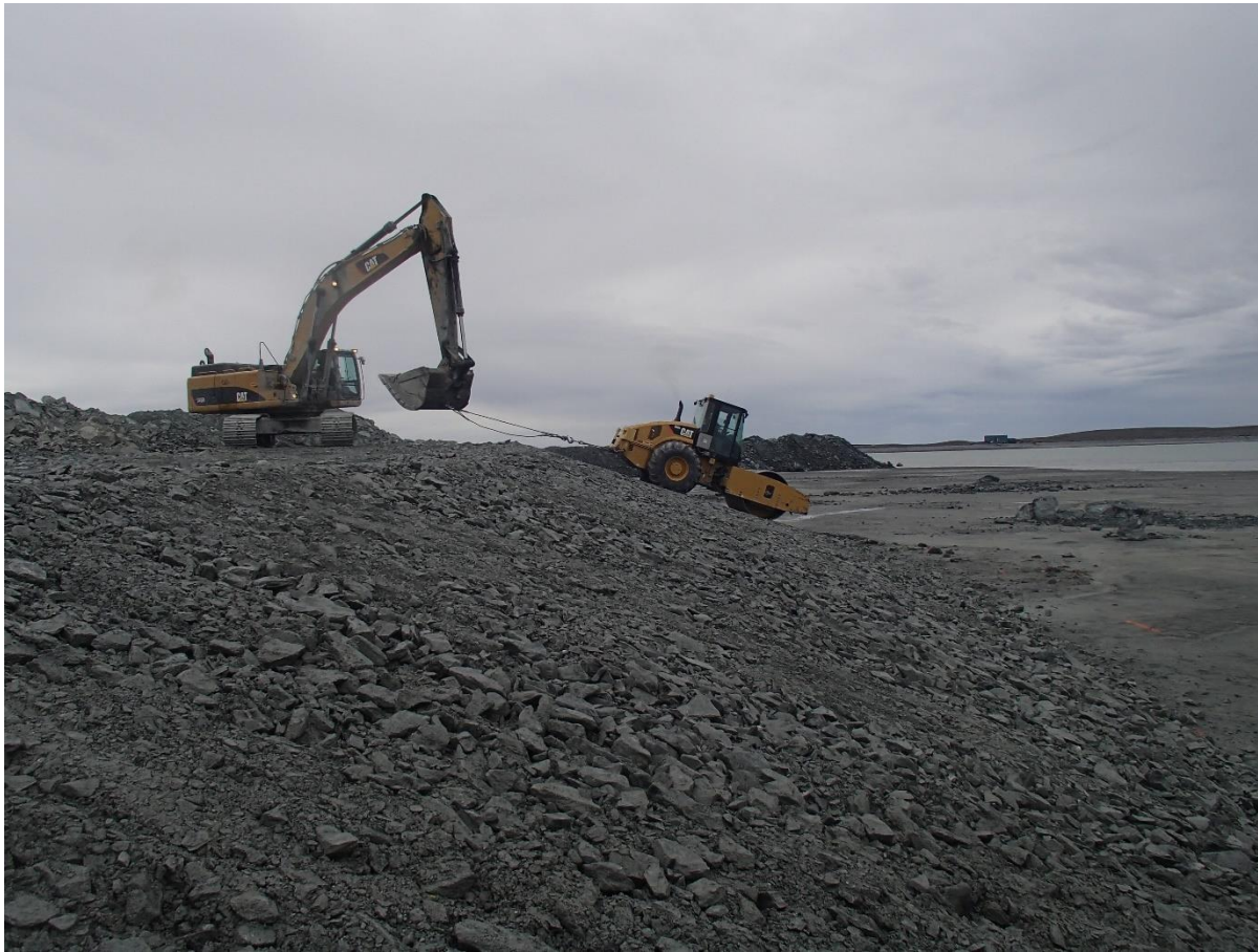
Photograph NCIS-080: From Sta. 2+800/-38 m (approx.), looking S. Compaction of the 0.5 m lift (approx.) of coarse filter between El. 150 and 152 m with a 10-tonne smooth-drum compactor (4 passes) in the upstream slope from Sta. 2+925 m to 3+160 m and from Sta. 1+300 m to 1+200 m.
