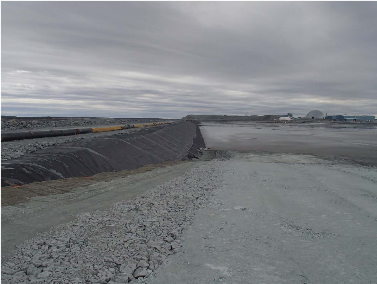
Photograph CD-1899: From Sta. 0+140/-33 m, looking S. View of Central Dike at the end of the 2018 construction phase.
