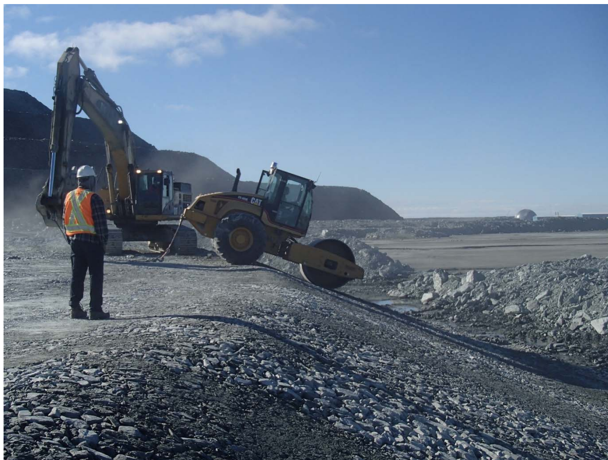
Photograph NCIS-054: From Sta. 2+580/-31 m (approx.), looking SE. Compaction of the 0.5 m lift (approx.) of coarse filter between El. 150 and 152 m with a 10-tonne smooth-drum compactor with vibration (4 passes) in the upstream slope from Sta. 2+560 m to 2+815 m.
