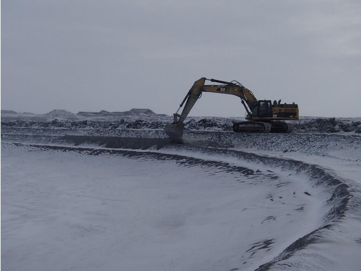
Photograph CD-1838: From Sta 40+750/-31 m, looking NE. Placement of a second 0.5 m thick lift of fine filter from El. 143.5 m to 144 m upstream of the coarse filter with an excavator from Sta. 0+500 m to 0+835 m and from 0+930 to 40+730 m.
