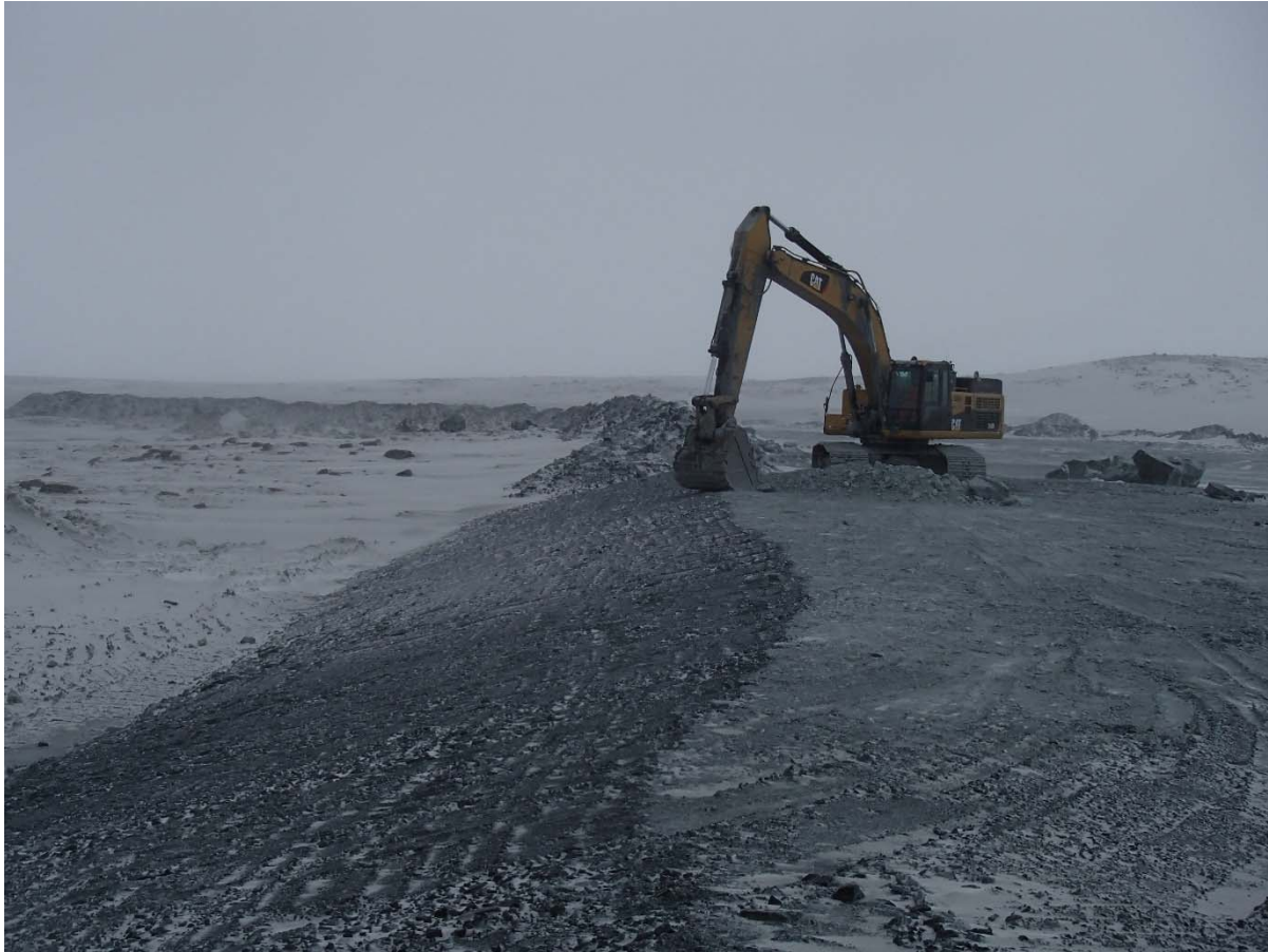
Photograph NCIS-019: From Sta. 2+100 m (approx.), looking SW. Profiling of the upstream slope (3H:1V) from El. 150 to 152 m with an excavator from Sta. 1+860 m to 1+678 m. The portion between Sta. 1+900 m and 1+800 m, where the structure is built on the natural ground, was not profiled.
