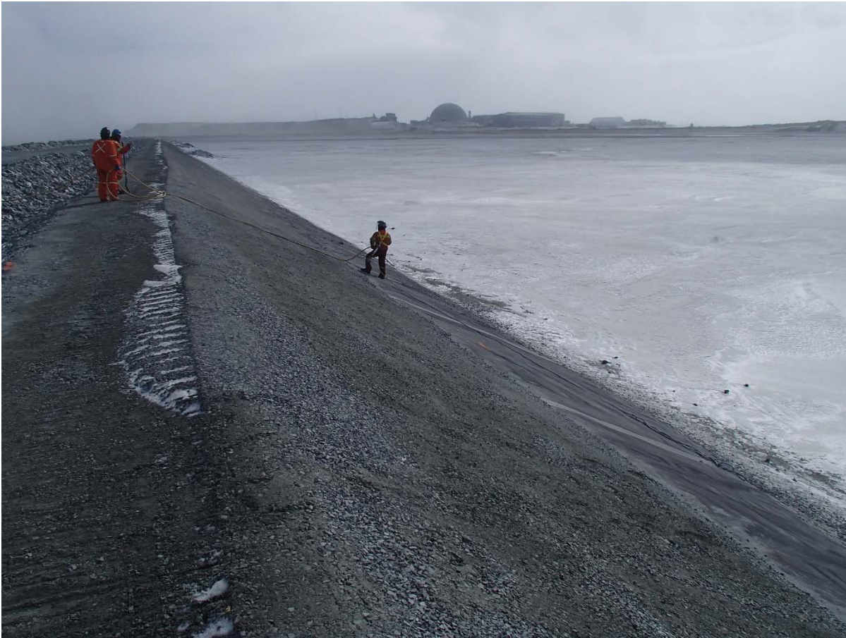
Photograph CD-1855: From Sta. 0+230/-22 m, looking S. Clean-up of the existing LLDPE with pressurized air stream in preparation for liner installation between Sta. 0+170 m and 40+780 m
