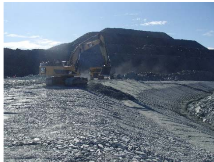
NCIS-104 (2018-07-21), looking SE from Sta. 2+650/-23 m (approx.). Placement of a 0.5 m thick lift of fine filter in the upstream slope from El. 152 m to 154 m with an excavator from Sta. 2+710 m to 2+445 m.
