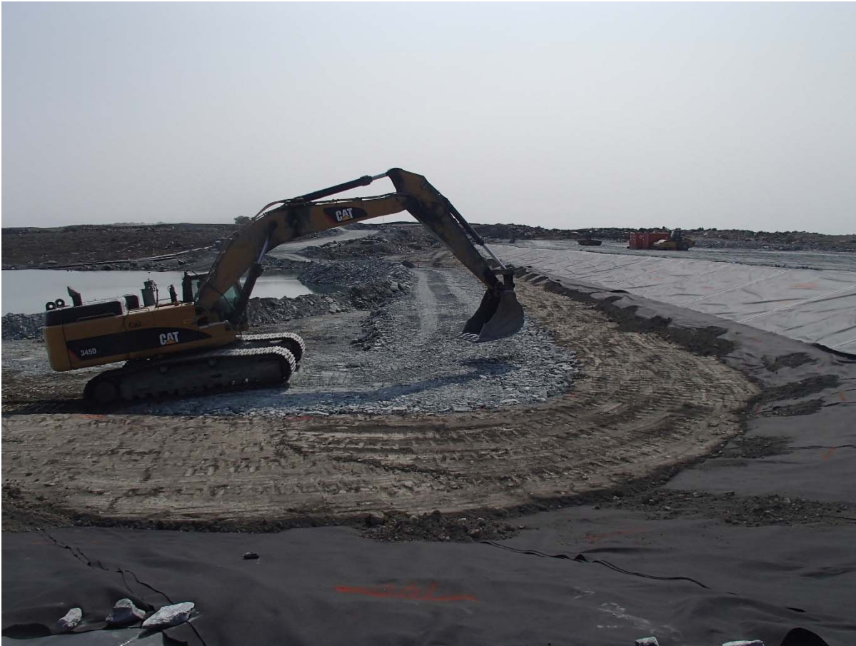
Photograph SD3-325: From Sta. 20+610/-43 m, looking S. Placement of a first 0.5 m thick lift of fine rockfill (0-500 mm) upstream of the low quality till from El. 142 m to 142.5 m from Sta. 20+610 m to 20+760 m.
