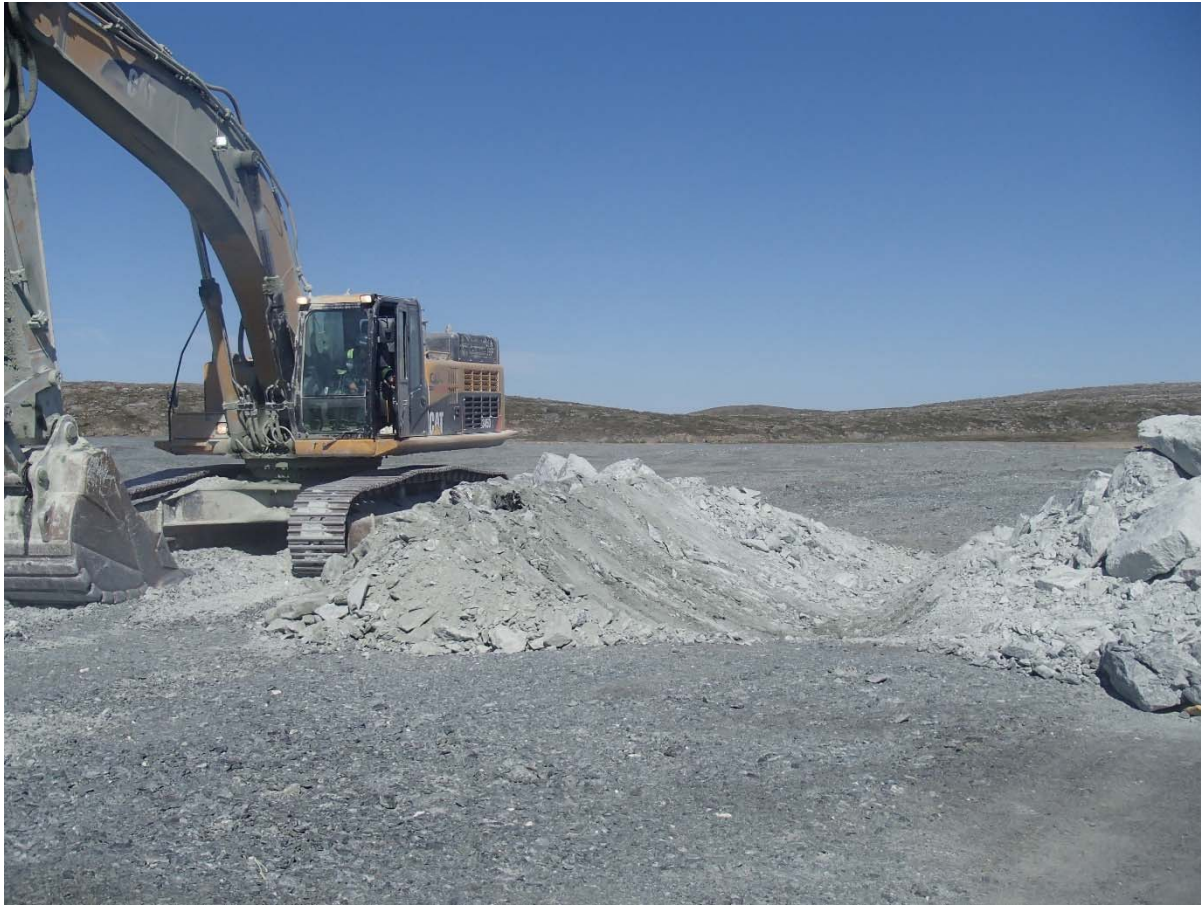
Photograph NCIS-114: From Sta. 1+700/-34 m (approx.), looking N. Excavation of a 0.8 m (approx.) deep, 1 m wide shallow ditch in the rockfill capping with an excavator from Sta. 1+500 m to 1+650 m.
