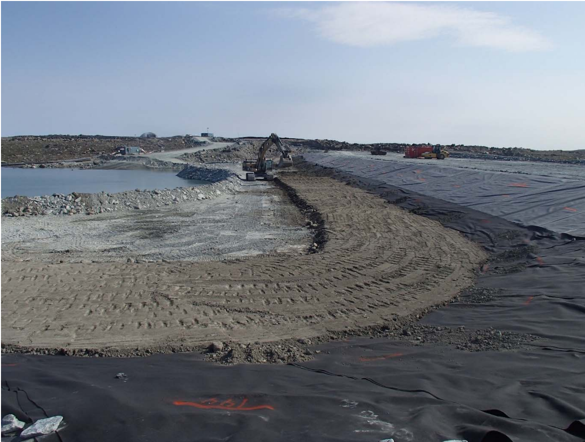
Photograph SD3-323: From Sta. 20+610/-43 m, looking S. Placement of the first lift of low quality till (0-150 mm) from El. 142 m to 142.5 m from Sta. 20+610 m to 20+715 m.
