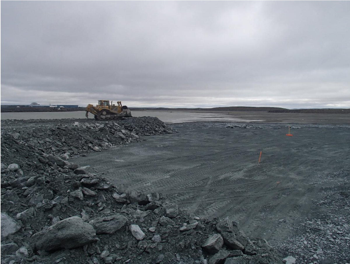
Photograph NCIS-082: From Sta 1+140/-52 m (approx.), looking SW. Placement of a 2 m thick (approx.) lift of IV rockfill from El. 150 m to El. 152 m (approx.) with a dozer from Sta. 1+160 m to 1+170 m (-64 m to -111 m). The material is of good quality and is well graded.
