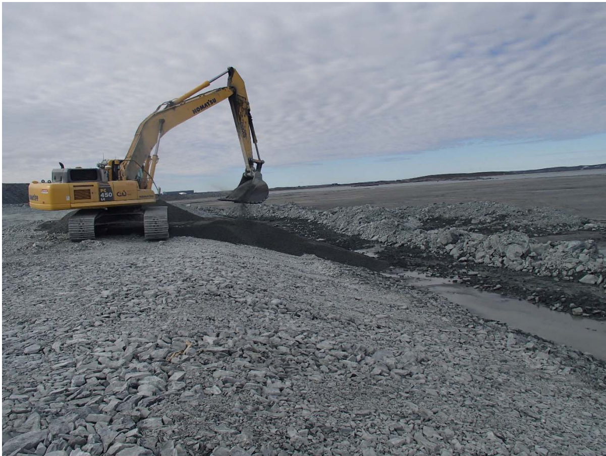
Photograph NCIS-036: From Sta. 1+900/-21 m (approx.), looking SE. Placement of a 0.5 m thick lift of fine filter over the coarse filter in the upstream slope from El. 150 m to 152 m with an excavator from Sta. 2+542 m to 2+475 m.
