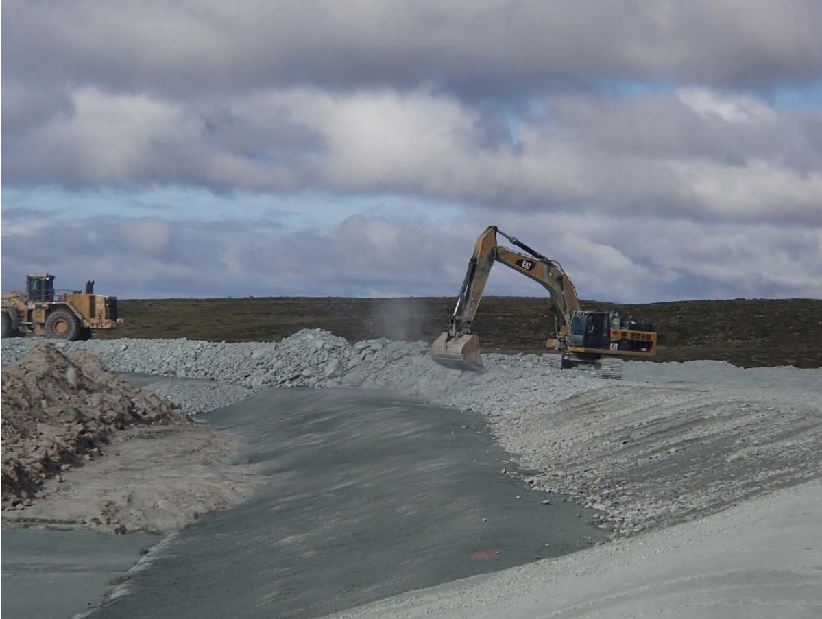
Photograph NCIS-132: From Sta. 1+940/-20 m (approx.), looking W. Profiling of the upstream slope (3H:1V) from El. 152 to 154 m with an excavator from Sta. 1+780 m to 1+660 m.
