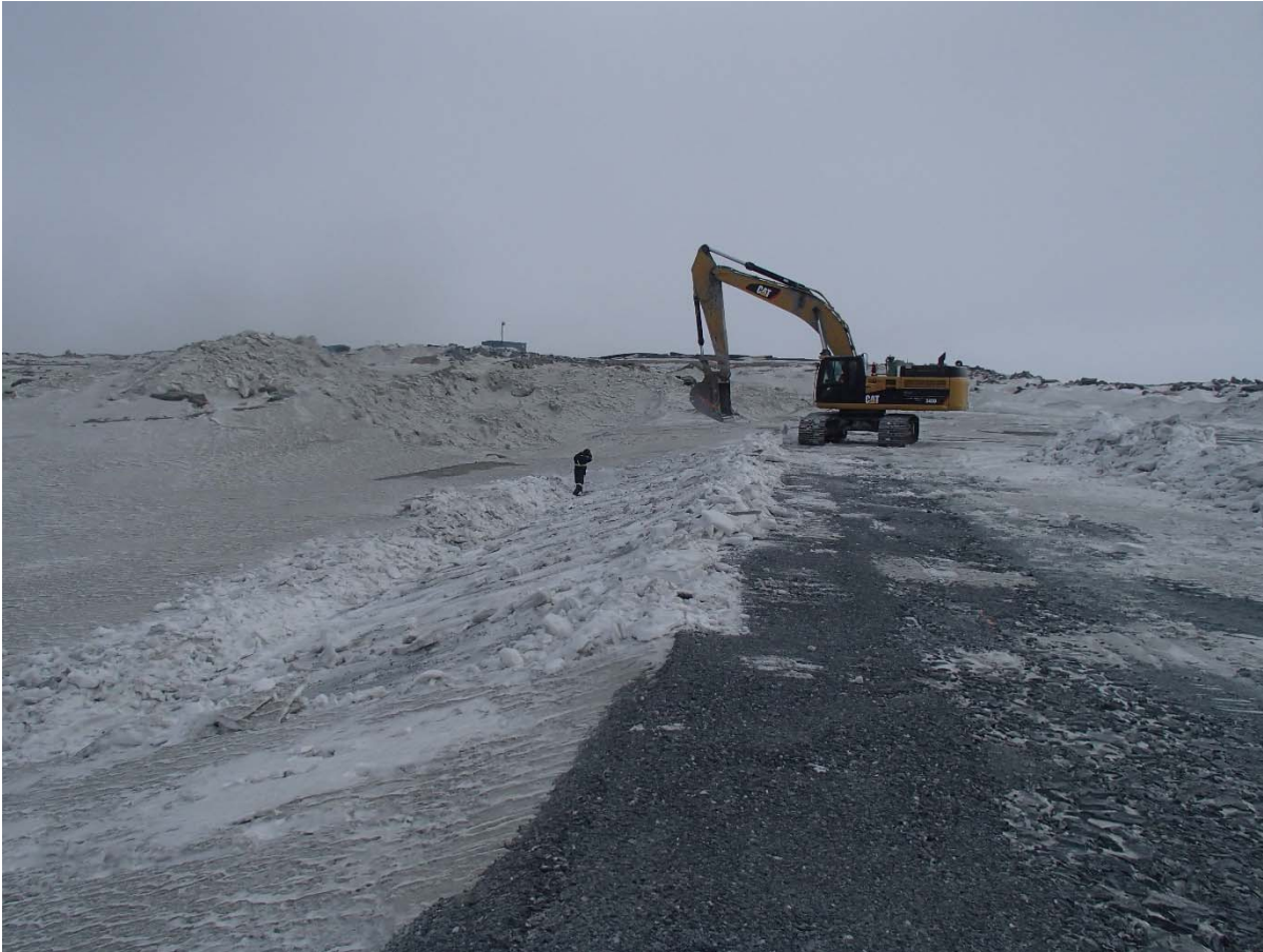
Photograph SD3-297: From Sta. 20+730/-10 m, looking SE. Removal of snow on the upstream slope of SD3 with an excavator, from Sta. 20+640 to 20+760 m.
