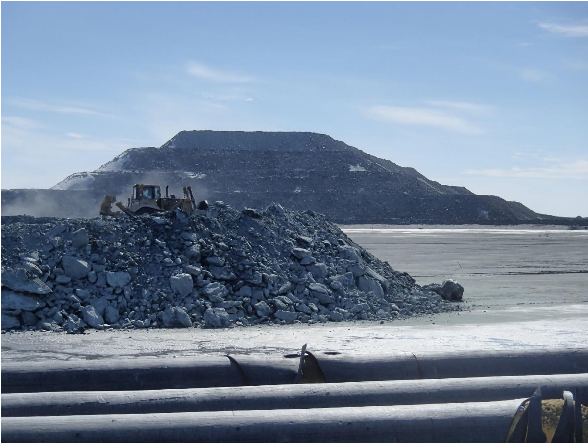
Photograph NCIS-027: From Sta. 1+360/+67 m, looking S. Placement of a 2 m thick (approx.) lift of UM rockfill from El. 150 m to El. 152 m (approx.) with a dozer from Sta. 1+365 m to 1+360 m (o.s. +9 m to -28 m).
