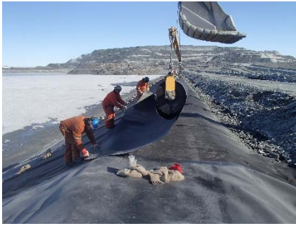
CD-1886 (2018-06-03), looking N from Sta. 0+485/-26 m. Installation of the LLDPE liner on the upstream slope 2H:1V between El. 143 m and 145 m from Sta. 0+480 m to 0+320 m (panel numbers 887 to 910).
