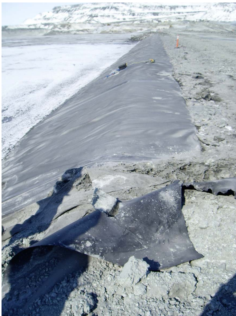
Photograph CD-1796: From Sta. 0+650/-28 m looking N. Damaged geomembrane near a deposition finger on Central Dike.
