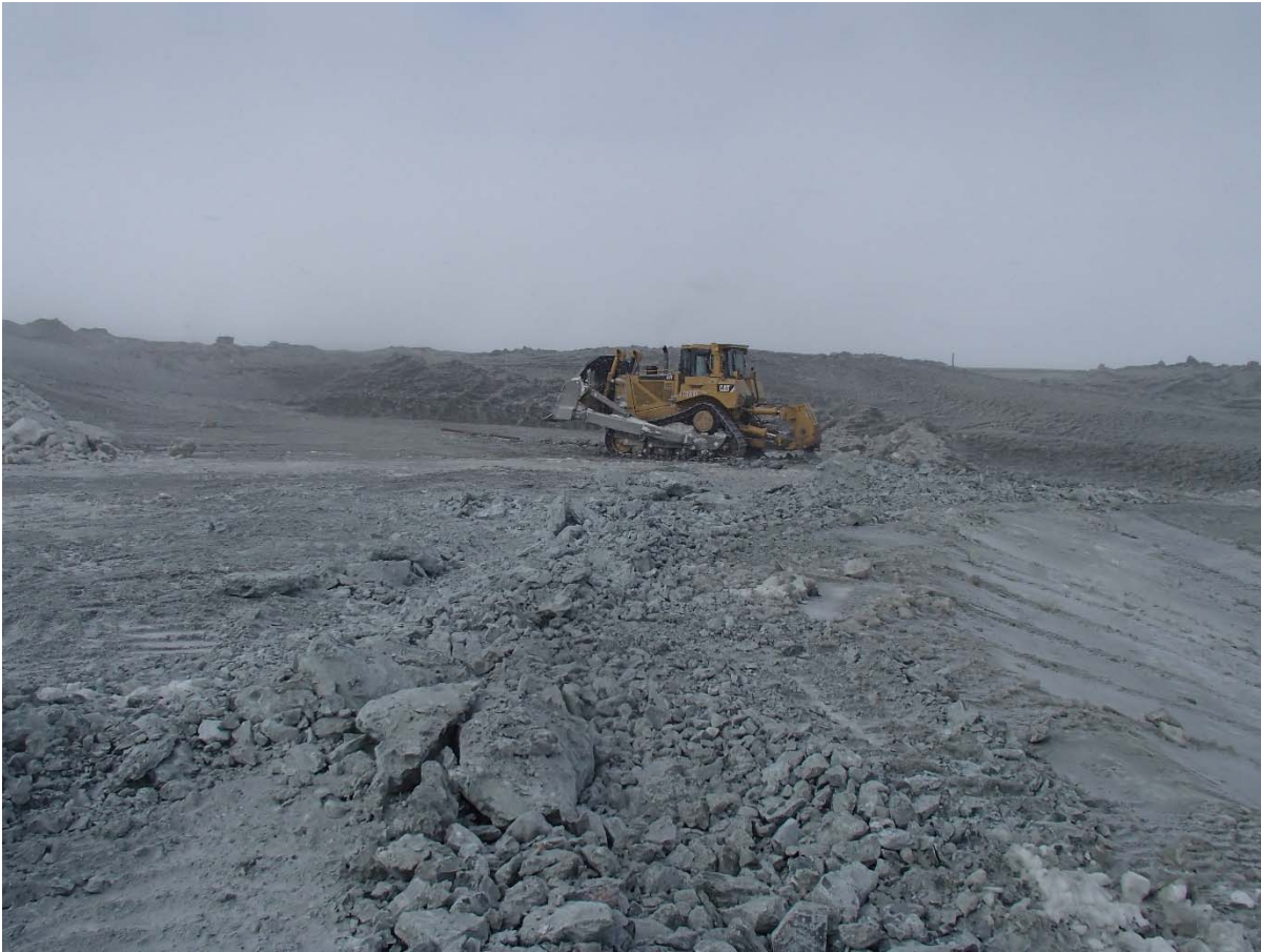
Photograph SD3-299: From Sta. 20+620/-26 m, looking NW. Scarification of the frozen ultramafic volcanic (UM) rockfill on the crest with a dozer for the anchoring trench excavation between Sta. 20+605 m and 20+780 m.
