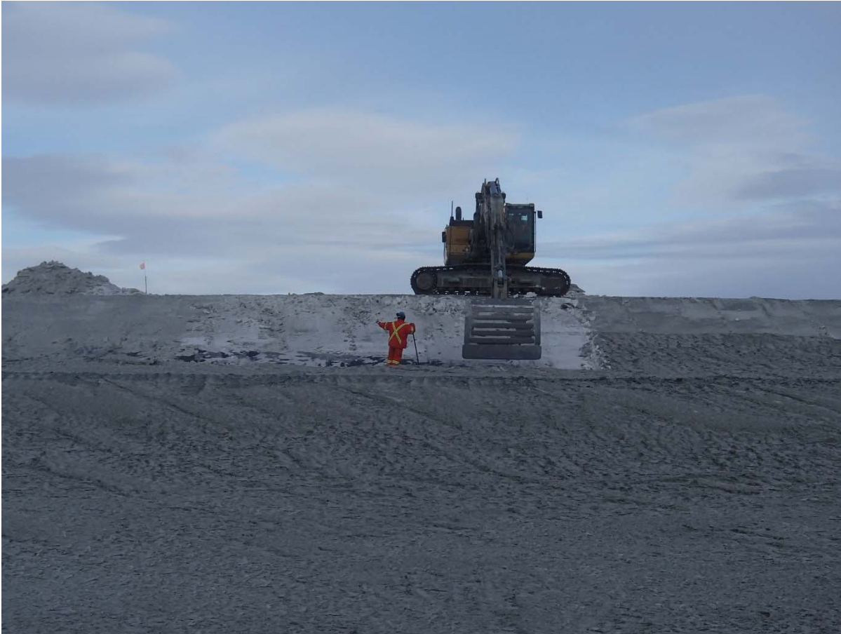
Photograph SD3-298: From Sta. 20+680/-88 m, looking S. Removal of snow on the upstream slope of SD3 above El. 142 m, from Sta. 20+620 m to 20+780 m.
