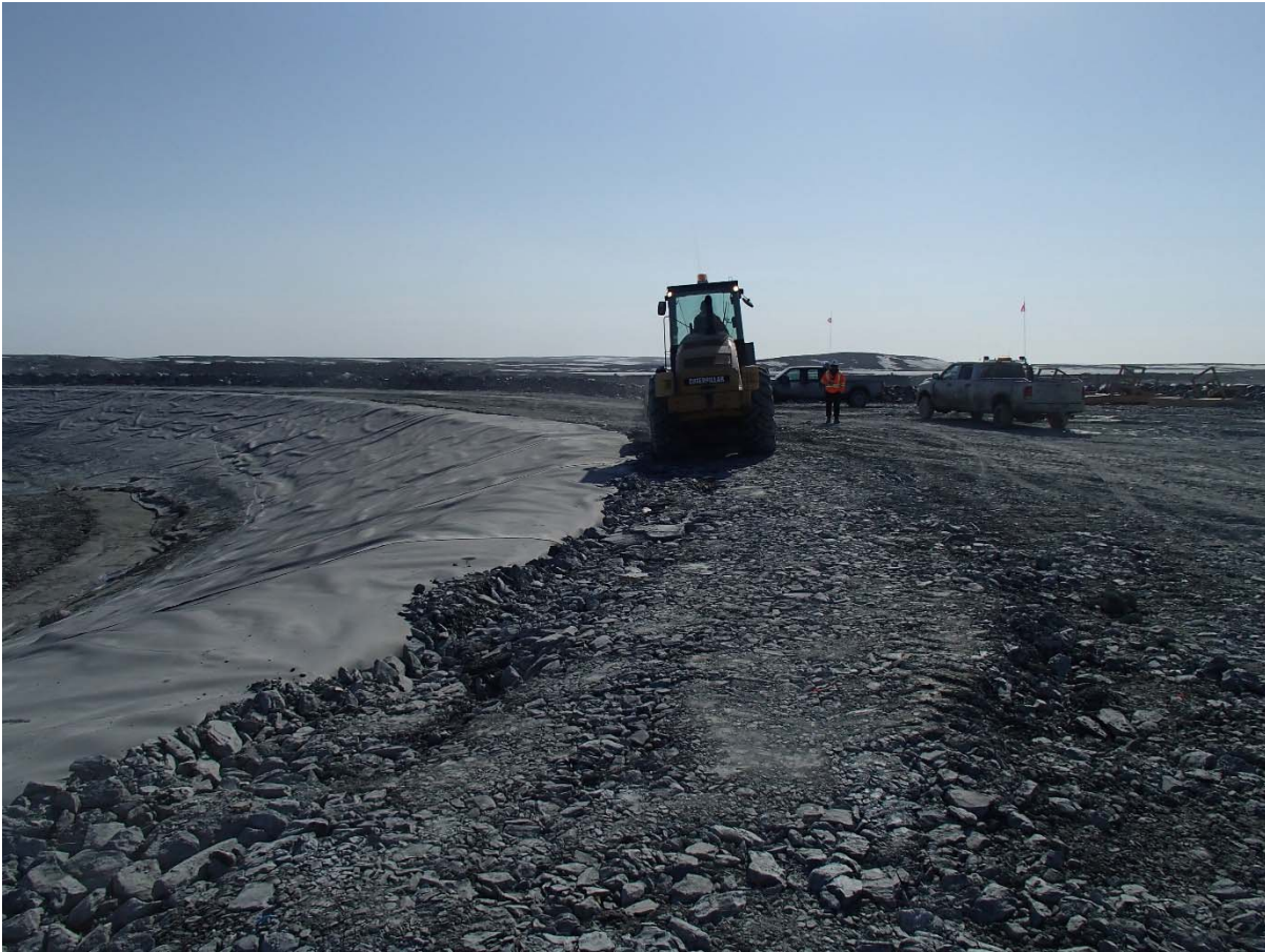
Photograph CD-1895: From Sta. 40+670/-15 m, looking E. Compaction of the geosynthetics tie-in material at El. 145 m with a 10-tonne smooth-drum compactor with vibration (4 passes) from Sta. 40+670 m to 0+950 m (approx.).
