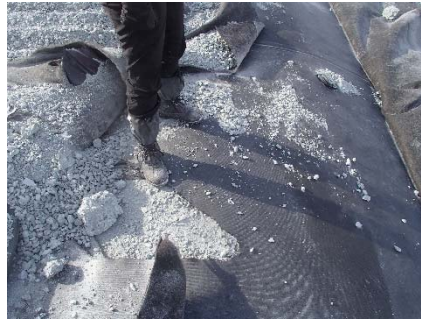
CD-1833 (2018-05-07), looking S from Sta. 0+390/-25 m. Damaged geomembrane near a deposition finger on Central Dike at Sta. 0+390 m.
