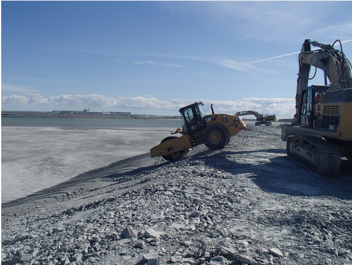
Photograph NCIS-099: From Sta. 1+180/-76 m (approx.), looking SE. Compaction of the 0.5 m lift (approx.) of coarse filter between El. 150 m and 152 m with a 10-tonne smooth-drum compactor with vibration (4 passes) in the upstream slope from Sta. 1+200 m to 1+170 m.
