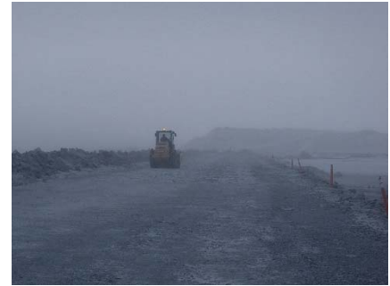
CD-1810 (2018-04-30), looking S from Sta. 0+335/-15 m. Compaction of the 2 m lift (approx.) of IV rockfill at El. 145 m with a 10-tonne smooth-drum compactor with vibration (6 passes) from Sta. 0+350 to 0+540 m (o.s. -19 to -7 m).
