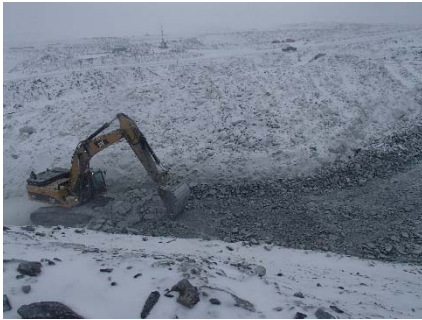
CD-1808 (2018-04-28), looking E from Sta. 40+790/-14 m. Placement a 2 m thick (approx.) lift of intermediate volcanic (IV) rockfill from approx. Sta. 40+780 to 40+805 m (o.s. -6 to 9 m).
