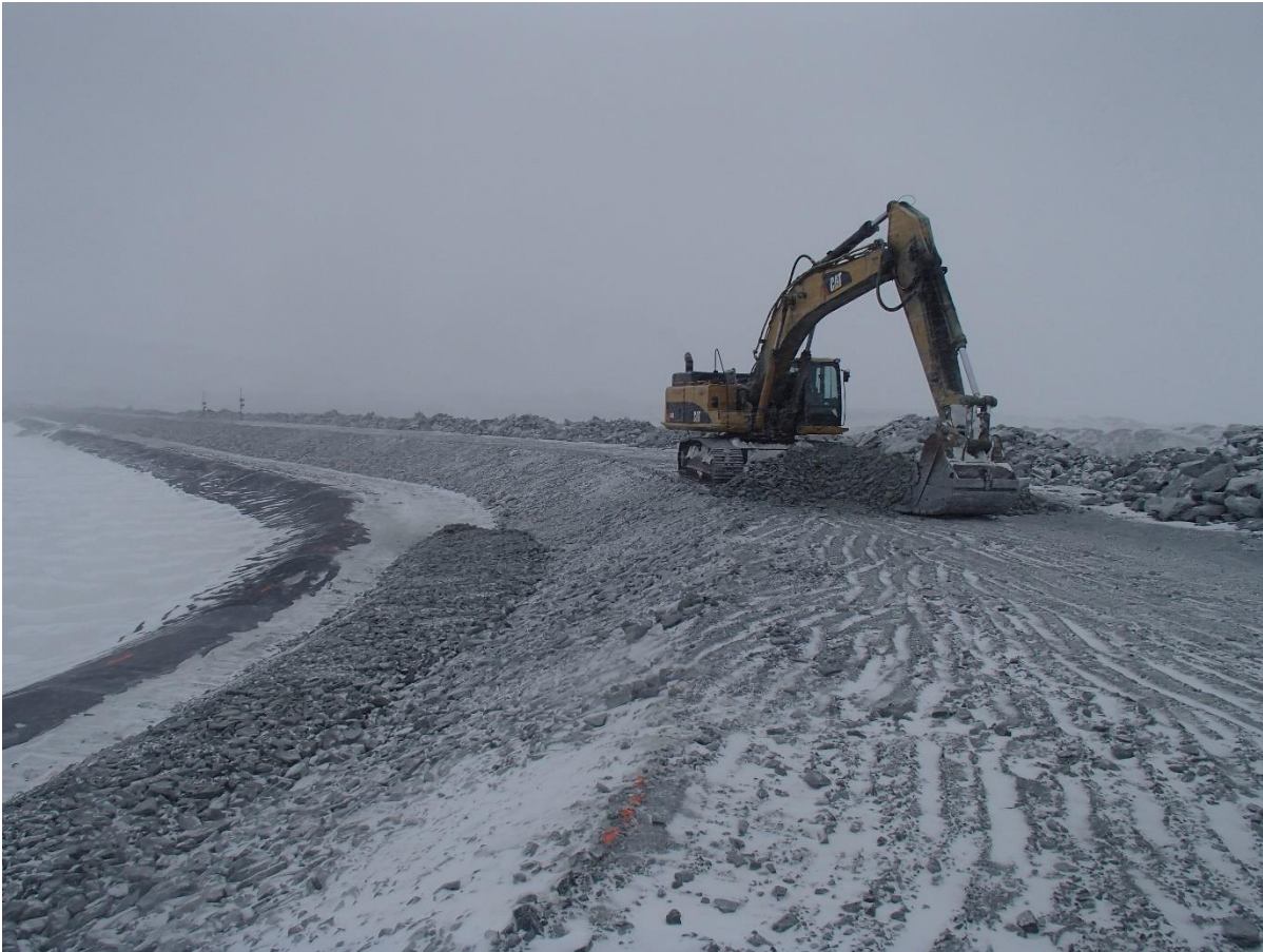
Photograph CD-1826: From Sta 40+770/-27 m, looking NE. Placement of a 0.5 m thick lift of coarse filter from El. 143 m to 143.5 m with an excavator from Sta. 40+730 m to 0+ 775 m.
