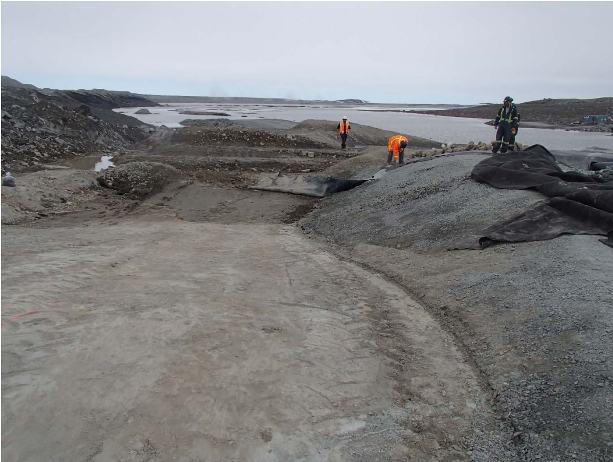
Photograph SD3-314: From Sta. 20+590/-32 m, looking E. View of the liner bedding ready for geosynthetics installation.
