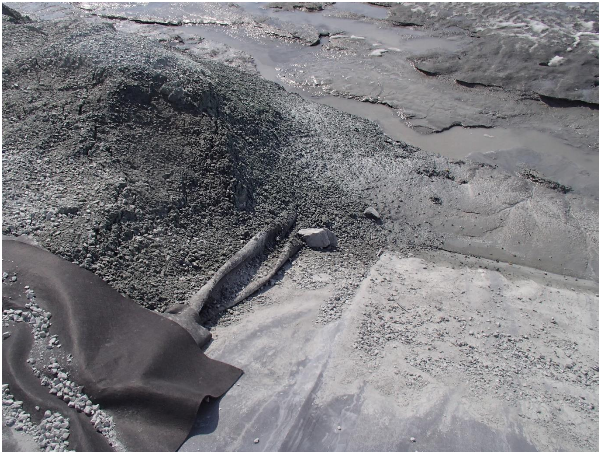
Photograph CD-1894: From Sta. 0+800/-28 m, looking E. View of a bloc in direct contact with the LLDPE liner following the construction of the deposition fingers on Central Dike.
