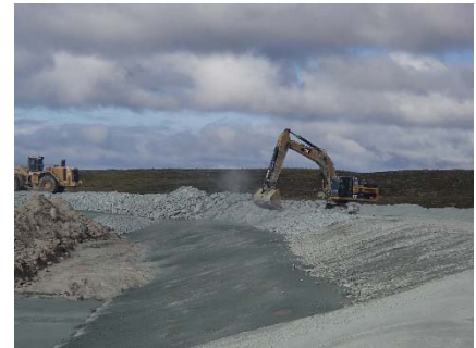
NCIS-132 (2018-07-29), looking W from Sta. 1+940/-20 m (approx.). Profiling of the upstream slope (3H:1V) from El. 152 to 154 m with an excavator from Sta. 1+780 m to 1+660 m.
