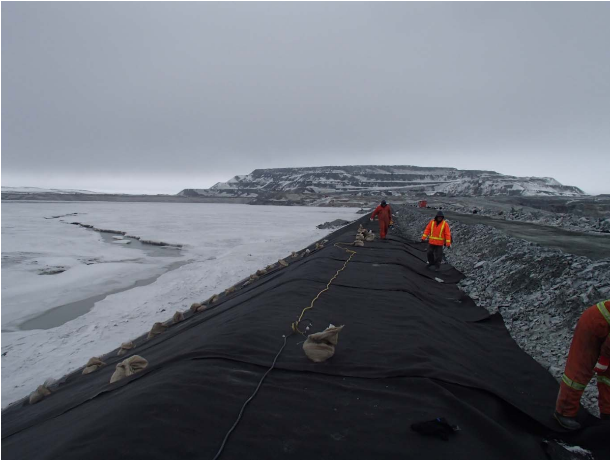
Photograph CD-1873: From Sta. 0+760/-26 m, looking N. Installation of the geotextile on the upstream slope 2H:1V between El. 143 m and 145 m from Sta. 0+760 m to 0+740 m.
