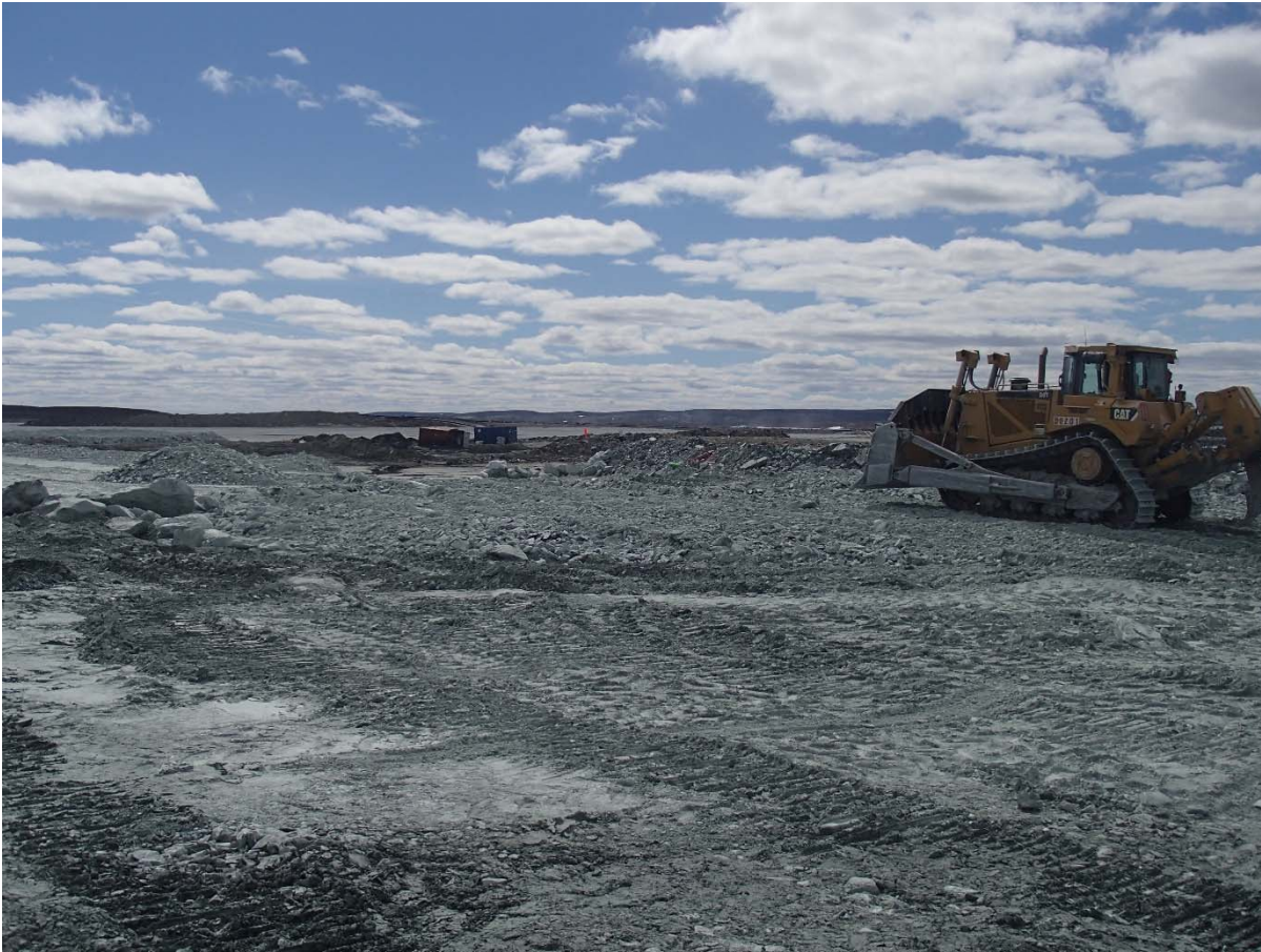
Photograph NCIS-060: From Sta. 1+365/-35 m (approx.), looking SW. Placement of a 2 m thick (approx.) lift of UM rockfill from El. 150 m to El. 152 m (approx.) with a dozer from Sta. 1+340 m to 1+320 m (-19 m to +16 m). The material is of good quality and is well graded.
