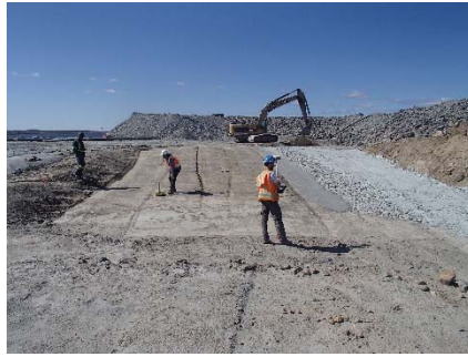
SD3-342 (2018-07-15), looking W from Sta. 20+600/-58 m. View of the compaction test and view of the filling of the depression between SD2 and SD3 with low quality till up to El. 145 m.
