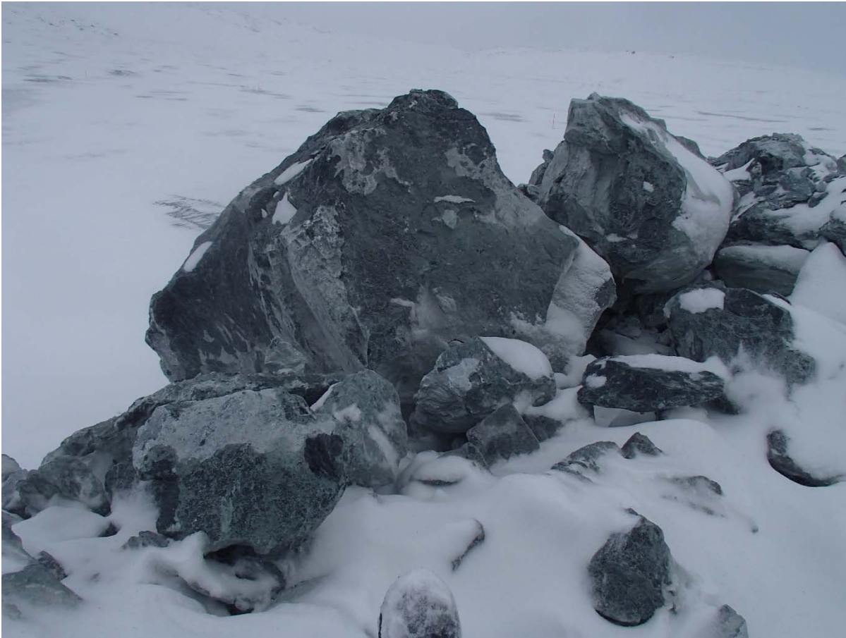
Photograph NCIS-006: View of oversize boulders on the UM rockfill lift at El. 152 m.
