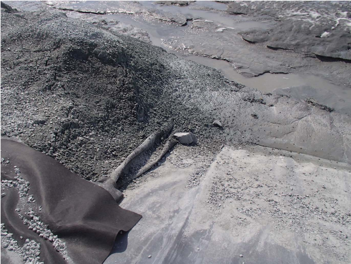
Photograph CD-1894: From Sta. 0+800/-28 m, looking E. View of a rock in direct contact with the LLDPE liner following the construction of the deposition fingers on Central Dike.
