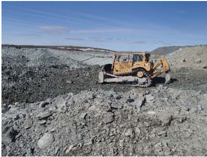
NCIS-049 (2018-06-26), looking N from Sta. 2+870/-28 m. Removing of UM rockfill material from the capping with a dozer to level the surface to El. 150 m from Sta. 2+760 m to 2+850 m (o.s. -29 to -17 m).
