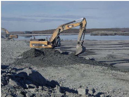
NCIS-076 (2018-07-04), looking SW from Sta. 2+940/-15 m. Placement of a 0.5 m thick lift of coarse filter in the upstream slope from El. 150 m to 152 m with an excavator from Sta. 2+980 m to 3+160 m.
