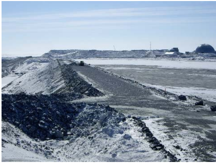
CD-1799 (2018-04-24), looking S from Sta. 0+080/-25 m. Placement a 2 m thick (approx.) lift of intermediate volcanic rockfill from El. 143 m to El. 145 m from 0+340 to 0+435 m (o.s. -28 to -18 m).
