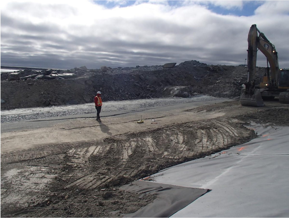
Photograph SD3-334: From Sta. 20+780/-26 m, looking SE. Compaction of the second 0.5 m thick lift of compacted sieved till and third lift of fine filter, coarse filter and fine rockfill of the upstream toe liner tie-in with a 10 tonne smooth-drum compactor with vibrations from Sta. 20+770 m to 20+800 m.
