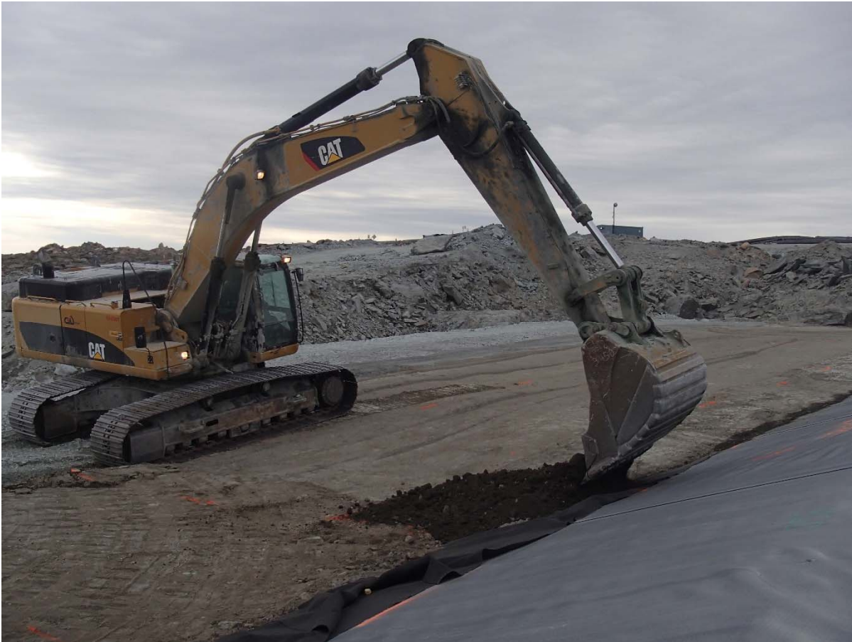
Photograph SD3-348: From Sta. 20+760/-25 m, looking E. Placement of a 0.5 m thick layer of compacted sieved till on the upstream slope of SD3 with an excavator from Sta. 20+777 m to 20+807 m. No large rock was allowed to be placed against the LLDPE liner.
