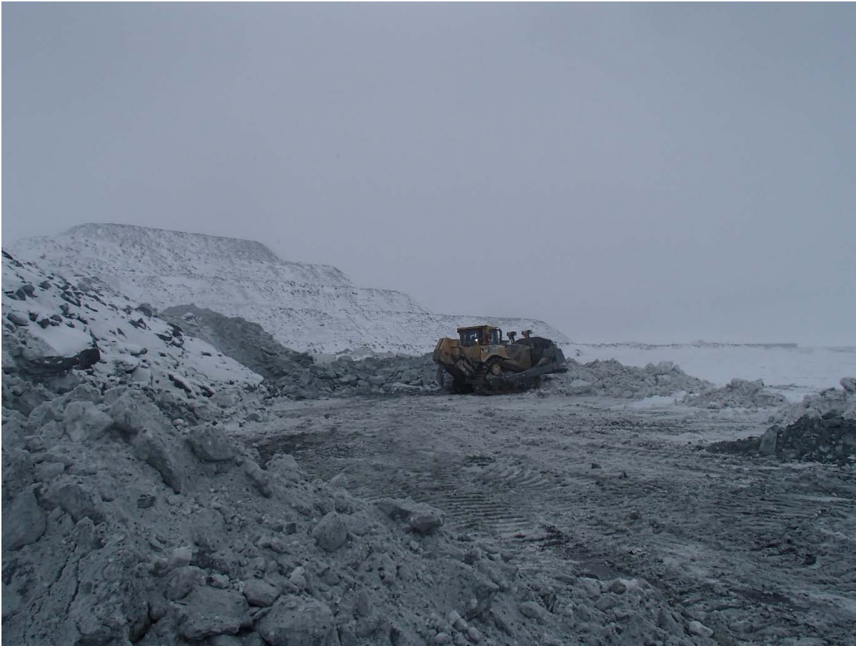
Photograph NCIS-005: Removal of the excavated material, pushed with a dozer towards the center of the North Cell to clear the upstream toe.
