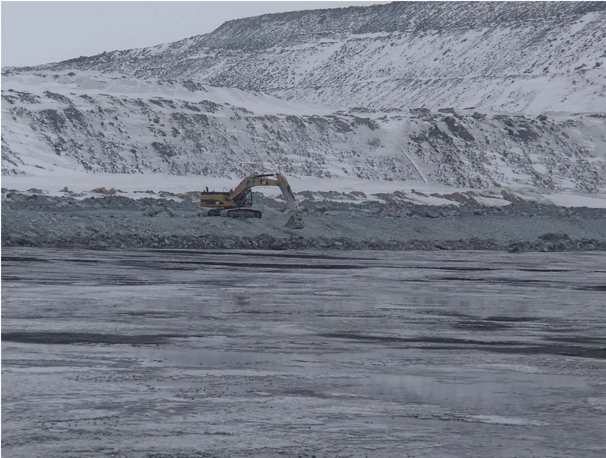
Photograph NCIS-010: Profiling of the upstream slope (3H:1V) from El. 150 to 152 m with an excavator from Sta. 2+777 m to 2+400 m (approx.).
