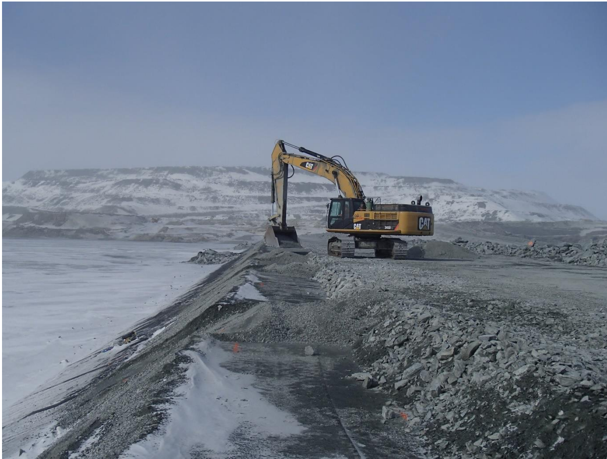
Photograph CD-1845: From Sta 0+660/-20 m, looking N. Profiling of the upstream slope (2H:1V) from El. 143 to 145 m with an excavator between Sta. 0+175 and 0+330 m and between Sta. 0+600 m and 0+715 m. The removed material is placed on the fourth 0.5 m thick lift of fine filter from El. 144.5 m to 145 m upstream of the coarse filter with an excavator from Sta. 0+170 m to 0+330 m and between Sta. 0+600 m and 0+715 m.
