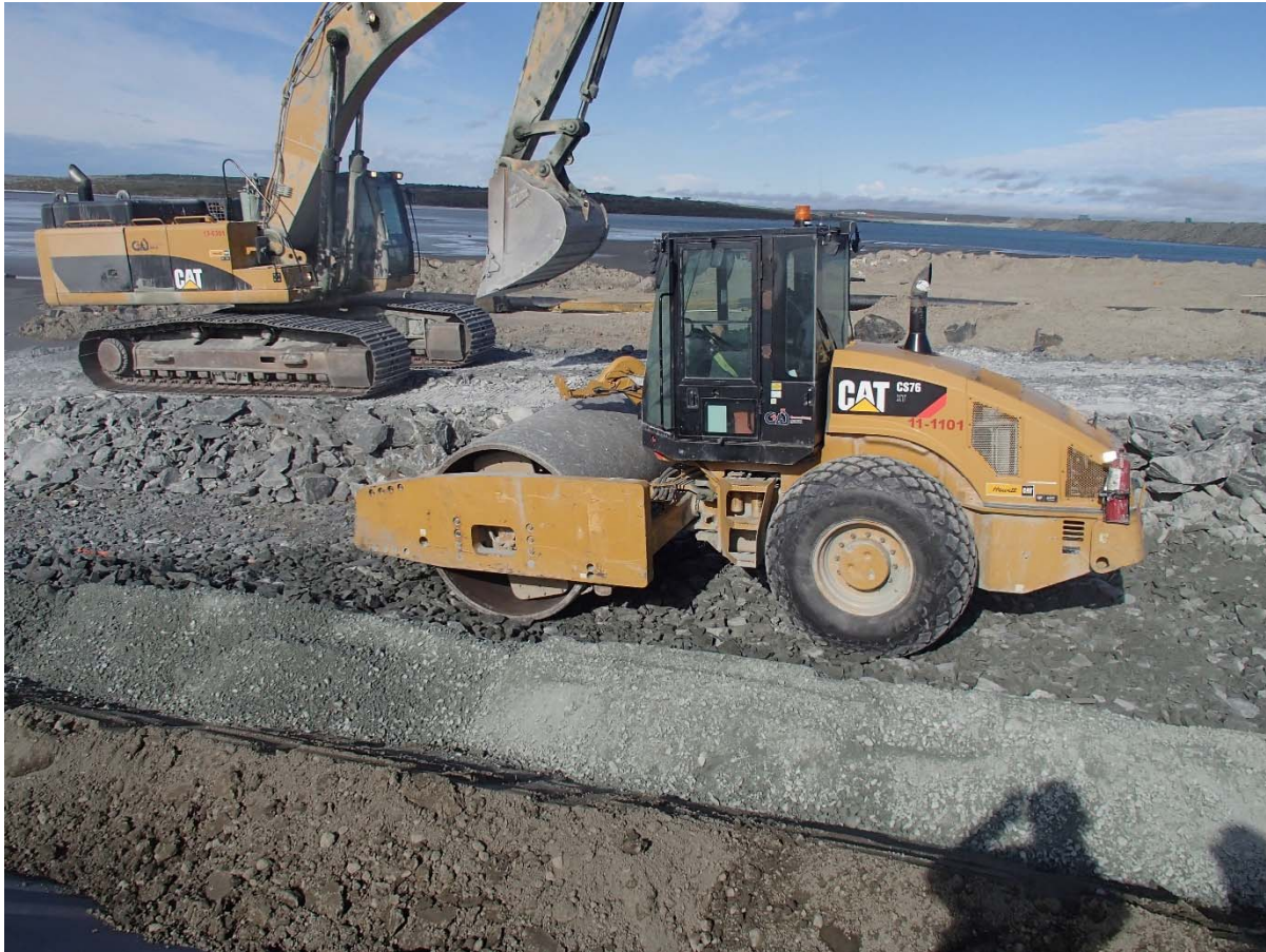
Photograph CD-1898: From Sta. 0+145/-30 m, looking W. Compaction of the 0.5 m thick lift of coarse filter on the top of the fine filter on the top of the upstream toe liner tie-in and on the upstream slope with a 10 tonne smooth-drum compactor with vibration (4 passes) from Sta. 0+147 m to 0+177 m.
