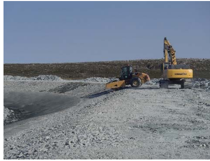
NCIS-110 (2018-07-23), looking N from Sta. 2+320/-22 m (approx.). Compaction of the 0.5 m lift (approx.) of coarse filter between El. 152 m and 154 m with a 10-tonne smooth-drum compactor with vibration (4 passes) in the upstream slope from Sta. 2+293 m to 2+080 m.
