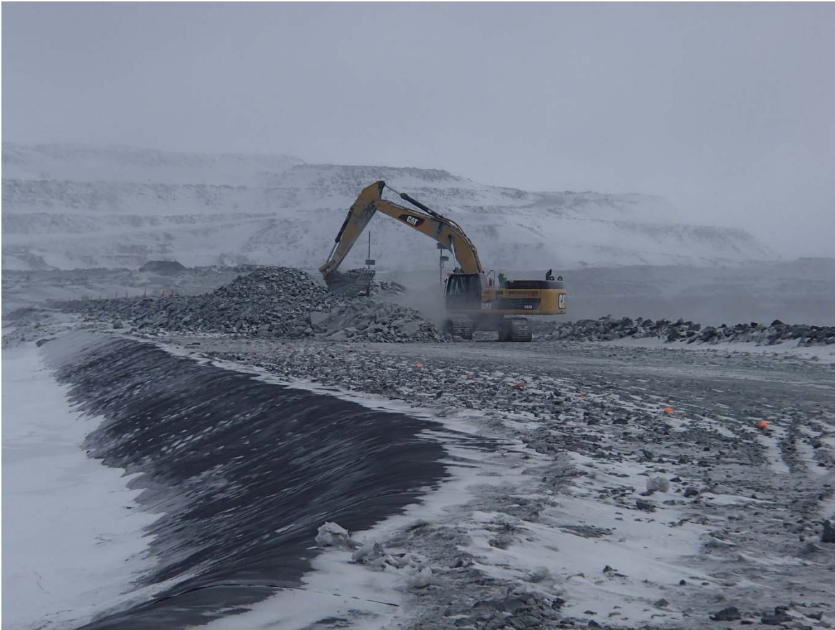
Photograph CD-1814: From Sta. 0+970/-10, looking NE. Placement of intermediate volcanic (IV) rockfill around the instruments at approx. Sta. 0+830 m with the excavator.
