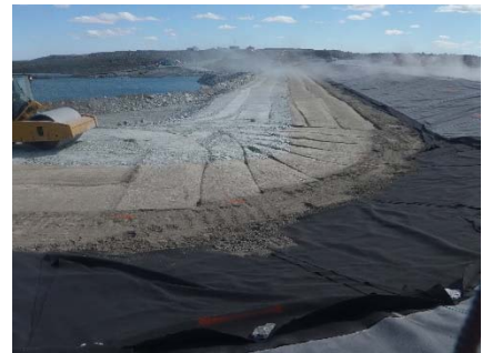
SD3-331 (2018-07-12), looking S from Sta. 20+610/-43 m. Compaction of the 0.5 m lift of low quality till (0-150 mm) at El. 143 m with a 10-tonne smooth-drum compactor with vibration (4 passes) from Sta. 20+610 m to 20+760 m.
