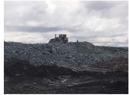
NCIS-084 (2018-07-08), looking E from Sta. 1+080/+47 m (approx.). Placement of a 2 m thick (approx.) lift of UM rockfill from El. 150 m to El. 152 m (approx.) with a dozer from Sta. 1+160 m to 1+130 m (-55 m to -102 m).
