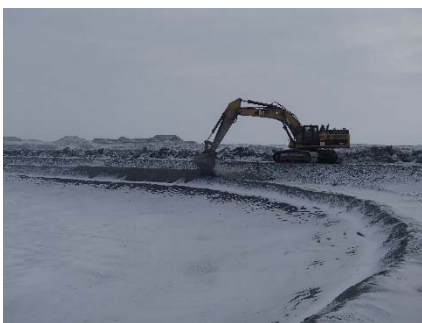
CD-1838 (2018-05-09), looking NE from Sta. 40+750/-31 m. Placement of a second 0.5 m thick lift of fine filter from El. 143.5 m to 144 m upstream of the coarse filter with an excavator from Sta. 0+500 m to 0+835 m and from 0+930 to 40+730 m.
