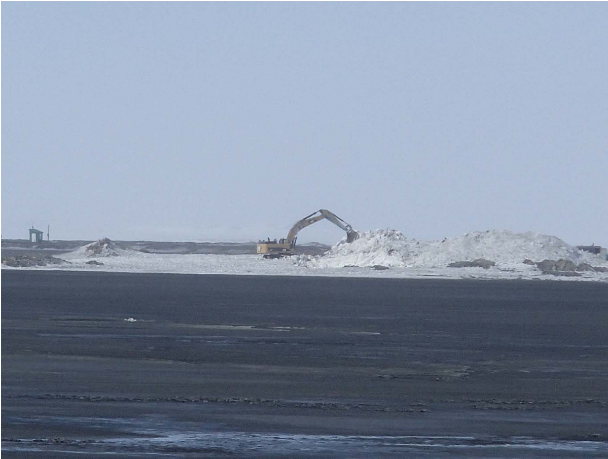
Photograph NCIS-024: From Sta. 2+570 m (approx.), looking SW. Removal of the snow bank in the footprint with an excavator from Sta. 1+160 m to 1+120 m (approx.).
