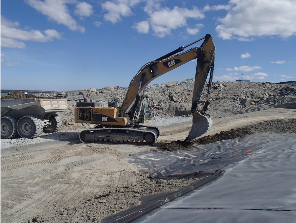
Photograph SD3-332: From Sta. 20+775/-23 m, looking SE. Placement of a first 0.5 m thick lift of compacted sieved till over the LLDPE geomembrane on the upstream toe liner tie-in with an excavator from Sta. 20+775 m to 20+800 m.
