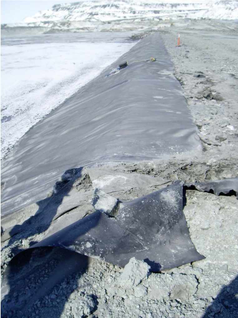
Photograph CD-1796: From Sta. 0+650/-28 m, looking N. Damaged geomembrane near a deposition finger on Central Dike.
