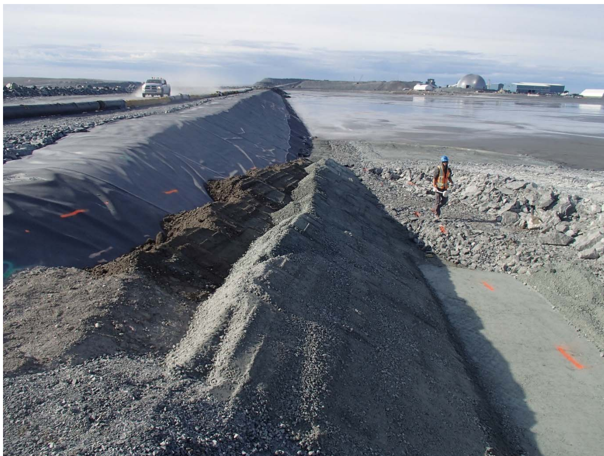
Photograph CD-1896: From Sta. 0+140/-30 m, looking S. Placement of 0.5 m thick layers of compacted sieved till and fine filter on the upstream slope of Central Dike with an excavator from Sta. 0+147 m to 0+177 m.
