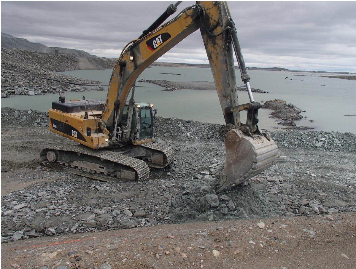
Photograph SD3-320: From Sta. 20+620/-67 m, looking E. Placement of a 1 m thick (approx.) lift of fine IV rockfill over the compacted till in the upstream slope from El. 142 m to 144 m with an excavator from Sta. 20+600 m to 20+610 m.
