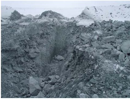
NCIS-001 (2018-05-19). View of a test pit in the UM rockfill lift at El. 152 m: a thick layer of snow (2 m) underlies the rockfill.
