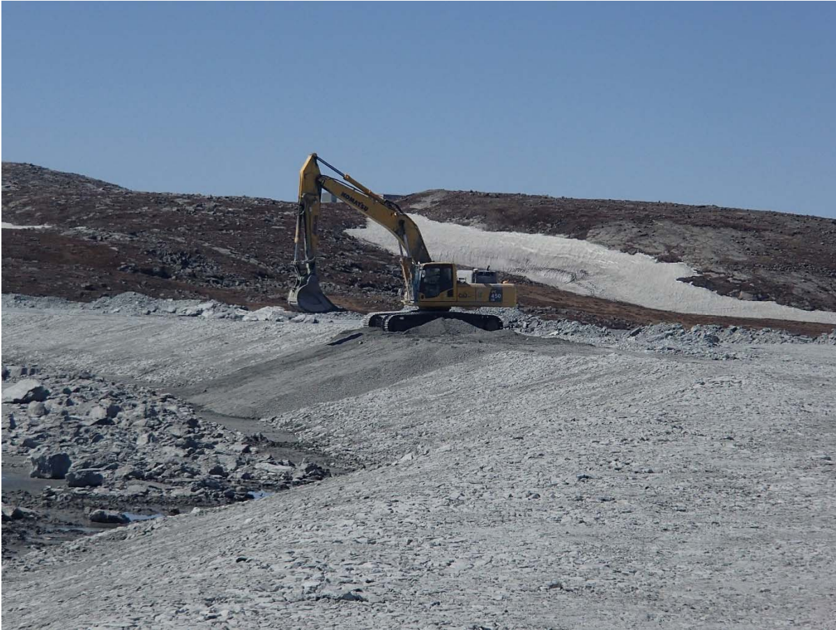
Photograph NCIS-039: From Sta. 2+200/-24 m (approx.), looking W. Placement of a 0.5 m thick lift of fine filter over the coarse filter in the upstream slope from El. 150 m to 152 m with an excavator from Sta. 2+460 m to 2+475 m and from Sta. 2+065 m to 1+980 m.
