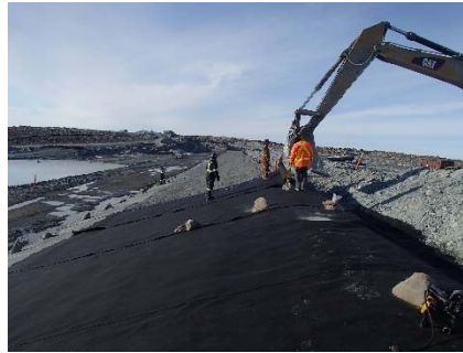
SD3-310 (2018-06-07), looking S from Sta. 20+635/-24 m. Installation of the geotextile on the upstream slope 3H:1V between El. 143 m and 145 m from Sta. 20+630 m to 20+800 m.
