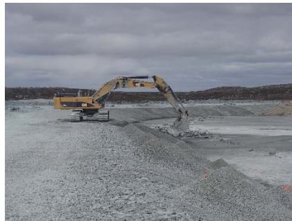
NCIS-062 (2018-06-29), looking N from Sta. 1+525/-33 m. Placement of a 0.5 m thick lift of fine filter over the coarse filter in the upstream slope from El. 150 m to 152 m with an excavator from Sta. 1+330 m to 1+260 m and from Sta. 1+595 m to 1+550 m.
