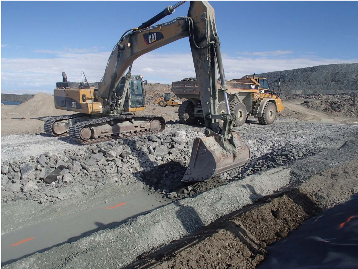
Photograph CD-1897: From Sta. 0+145/-30 m, looking NW. Placement of a 0.5 m thick lift of coarse filter on the top of the fine filter on the top of the upstream toe liner tie-in and on the upstream slope with an excavator from Sta. 0+147 m to 0+177 m.
