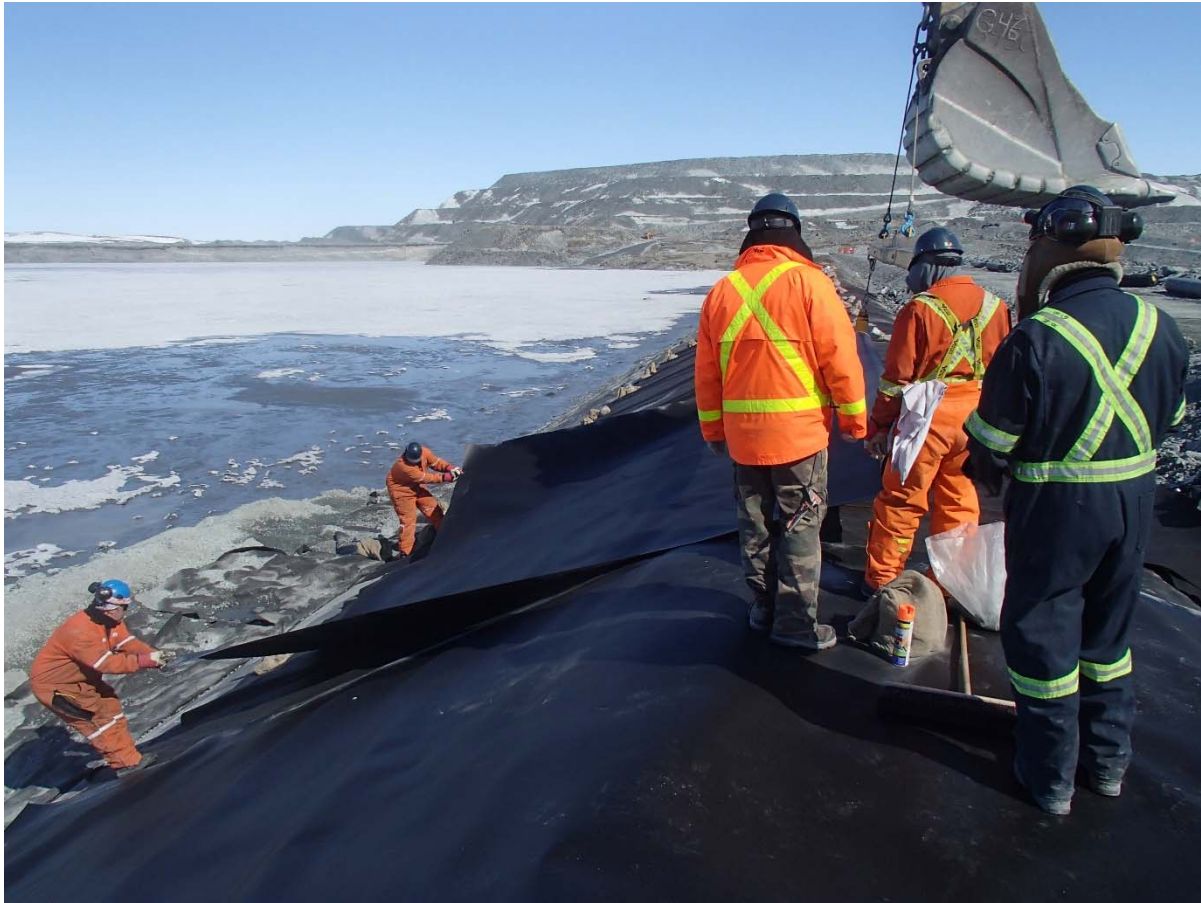
Photograph CD-1883: From Sta. 0+525/-26 m, looking N. Installation of the LLDPE liner on the upstream slope 2H:1V between El. 143 m and 145 m from Sta. 0+610 m to 0+480 m (panel numbers 868 to 886).
