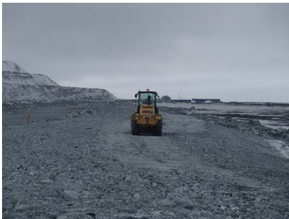
NCIS-022 (2018-05-30), looking SE from Sta. 2+245 m. Compaction of the 2 m lift (approx.) of ultramafic (UM) rockfill at El. 152 m with a 10-tonne smooth-drum compactor with vibration (6 passes) between the haul truck traffic lane and the upstream slope from Sta. 2+625 to 1+625 m (o.s. unavailable).
