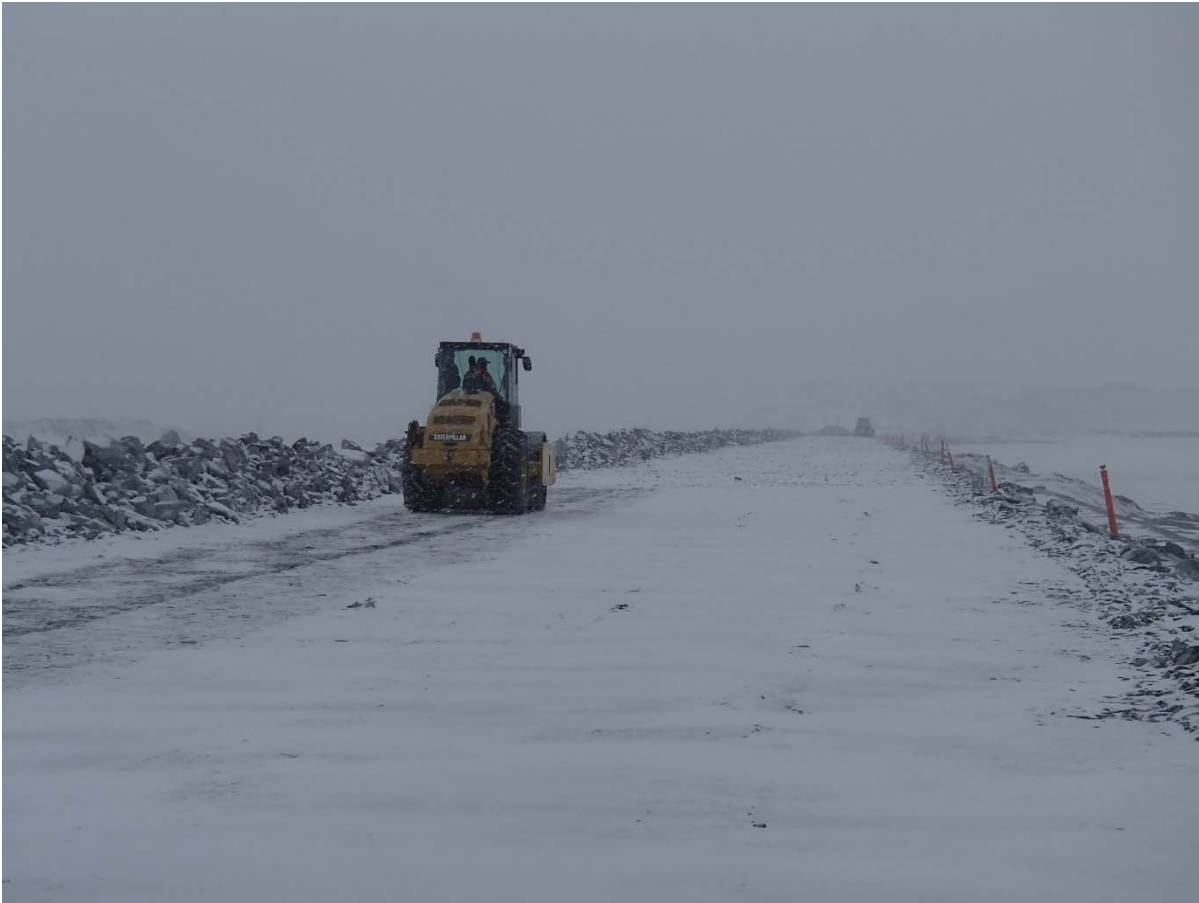
Photograph CD-1807: From Sta. 0+200/-15 m looking S. Compaction of the 2 m lift (approx.) of IV rockfill at El. 145 m with a 10-tonne smooth-drum compactor with vibration (6 passes) from Sta. 0+150 to 0+280 m (o.s. -21 to 11 m).
