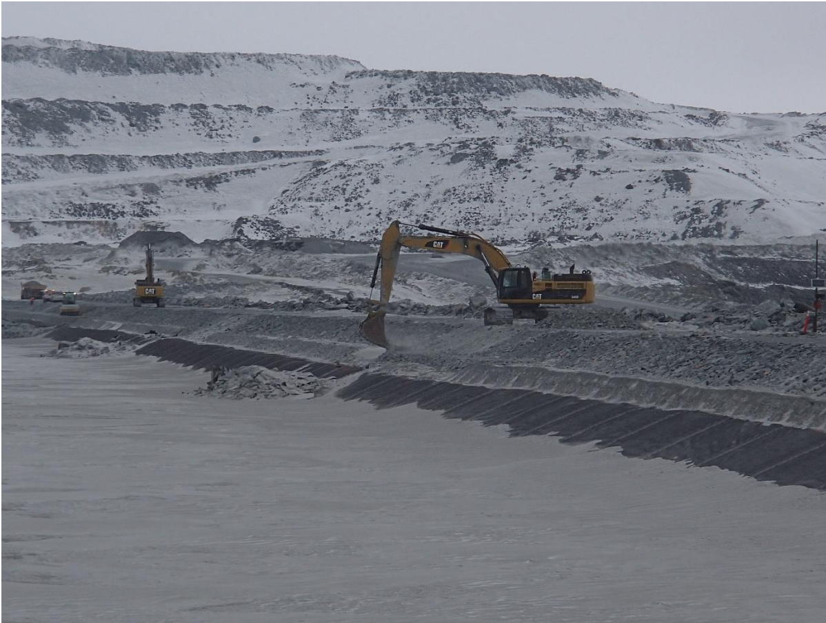
Photograph CD-1834: From Sta 40+760/-23 m, looking NE. Placement of a first 0.5 m thick lift of coarse filter from El. 143 m to 143.5 m on length of approx. 5 m with an excavator at the location of the deposition finger at Sta 0+520 m and 0+660 m.
