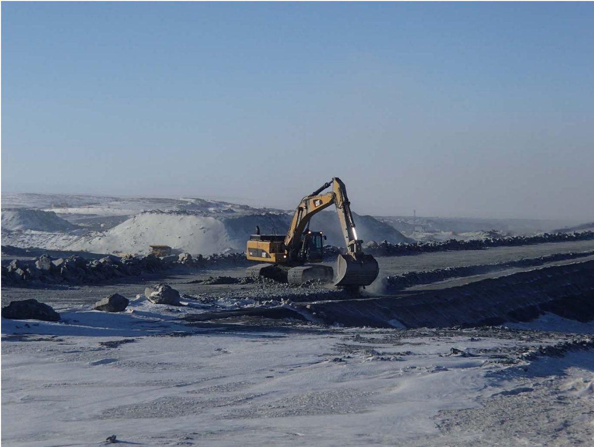
Photograph CD-1844: From Sta. 0+080/-49 m, looking SW. Placement of a fourth 0.5 m thick lift of coarse filter from El. 144.5 m to 145 m with an excavator from Sta. 0+170 m to 40+730 m.
