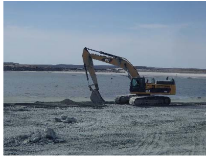
NCIS-068 (2018-07-01), looking S from Sta. 1+150/-62 m. Placement of a 0.5 m thick lift of fine filter over the coarse filter in the upstream slope from El. 148 m to 150 m with an excavator from Sta. 1+180 m to 1+100 m.
