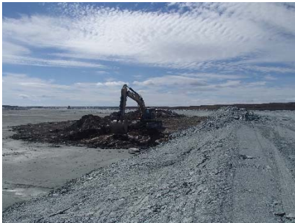
NCIS-031 (2018-06-20), looking SW from Sta. 1+880/-21 m. Final clean-up of the dike footprint with an excavator to reach a good quality bedrock from Sta. 1+800 to 1+850 m (o.s. -42 to -33 m).
