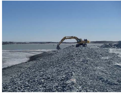
NCIS-092 (2018-07-14), looking S from Sta. 1+160/-77 m (approx.). Profiling of the upstream slope (3H:1V) from El. 150 to 152 m with an excavator from Sta. 1+185 m to 1+135 m.
