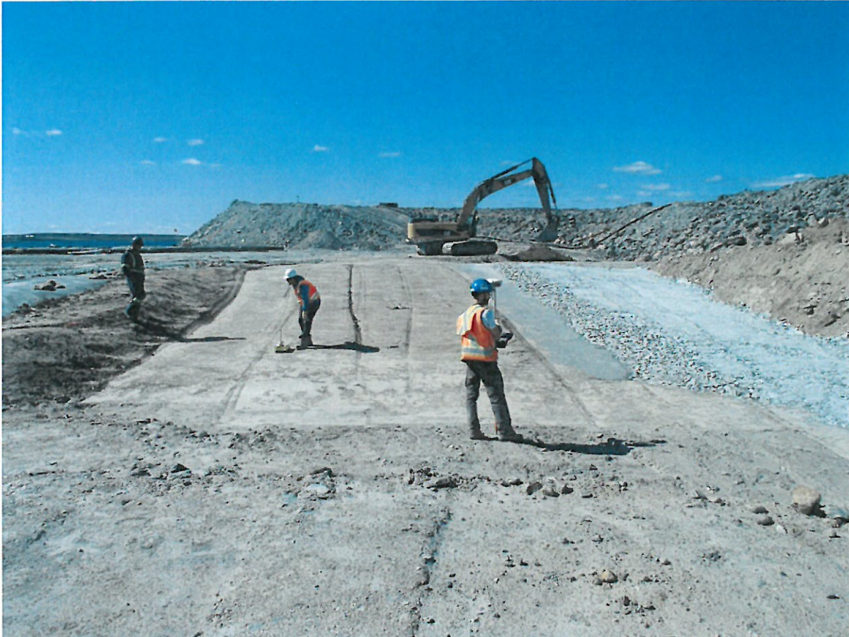
Photograph SD3-342: From Sta. 20+600/-57 m, looking W. View of the compaction test and view of the filling of the depression between SD2 and SD3 with low quality till up to El. 145 m
