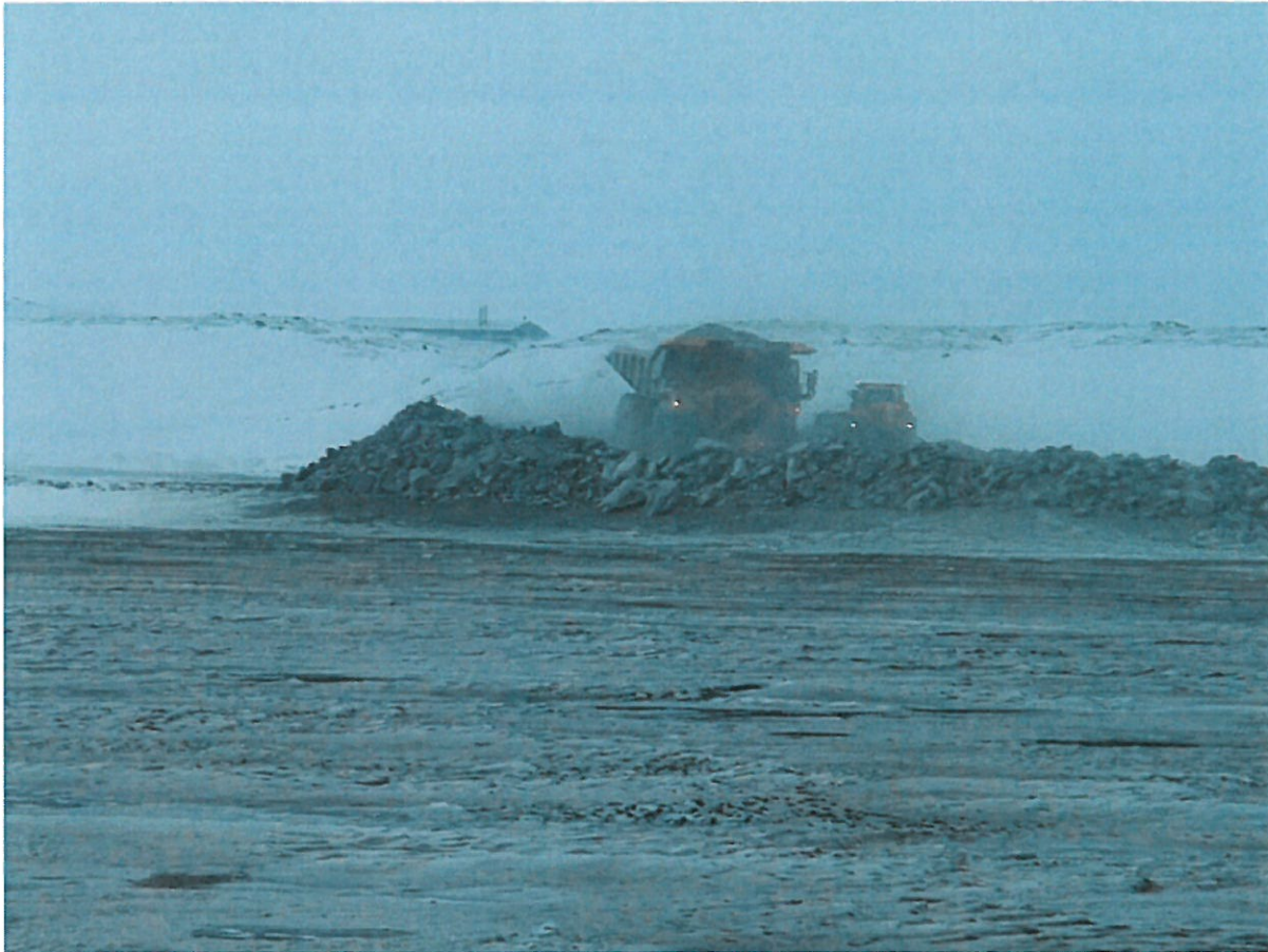
Photograph NCIS-008: Placement a 2 m thick (approx.) lift of UM rockfill from El. 150 m to El. 152 m (approx.) with a dozer. The material is of good quality and is well graded.
