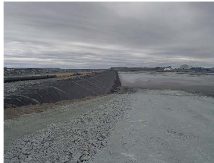
CD-1899 (2018-07-22), looking S from Sta. 0+140/-33 m. View of Central Dike at the end of the 2018 construction phase.
