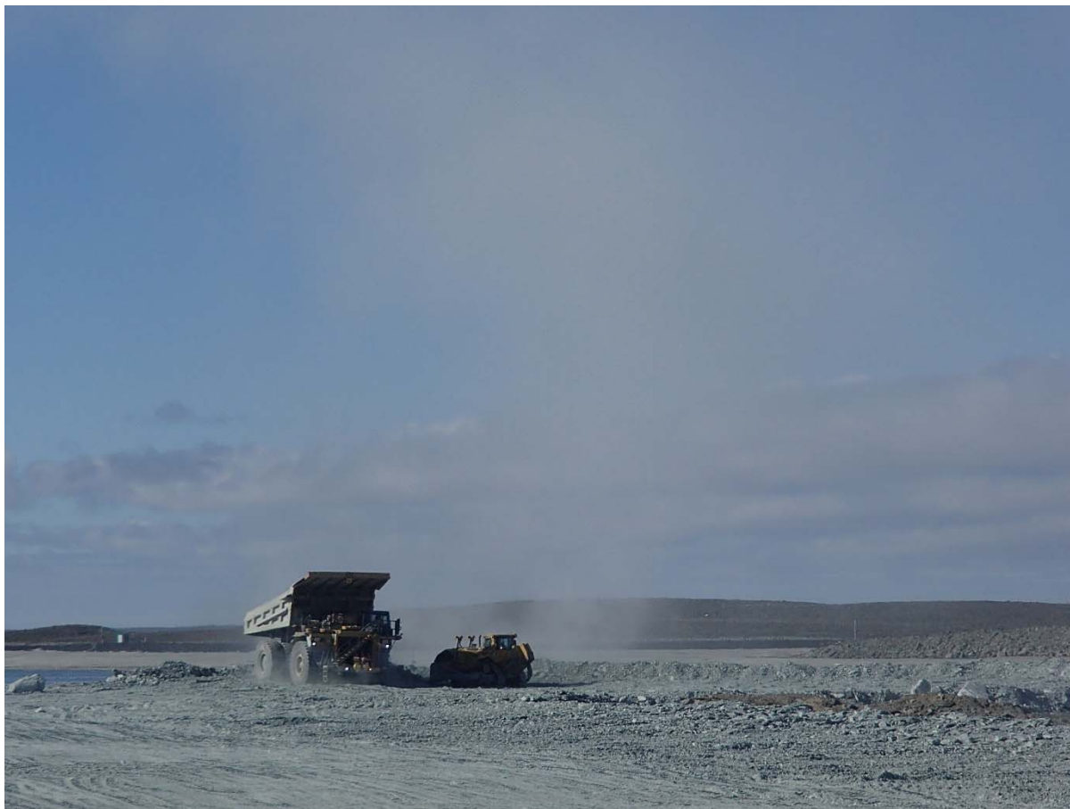
Photograph NCIS-059: From Sta. 1+330/-34 m (approx.), looking S. Placement of a 1.5 to 2 m thick (approx.) lift of UM rockfill from El. 148 m to El. 150 m (approx.) with a dozer from Sta. 1+120 m to 1+100 m (-96 m to -60 m). The material is of good quality and is well graded.
