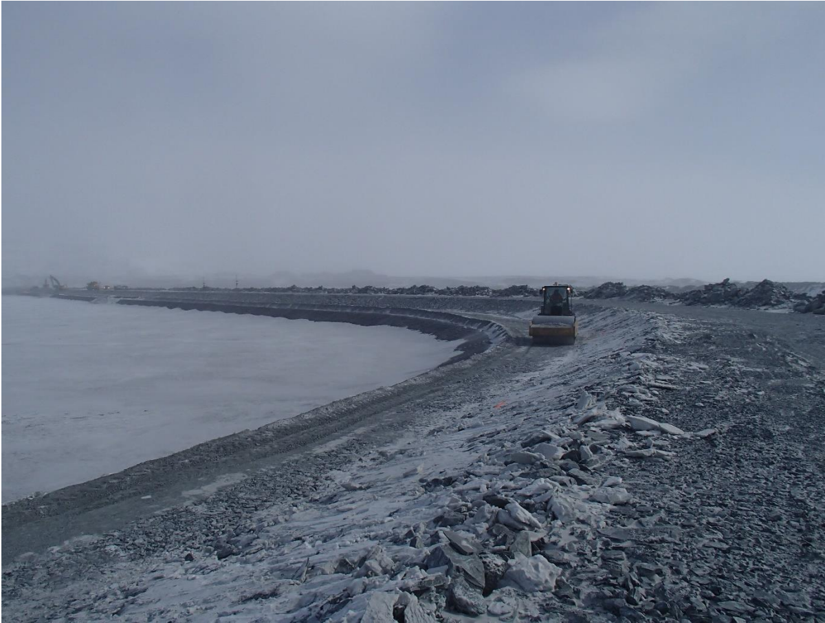
Photograph CD-1831: From Sta 40+730/-24 m, looking NE. Compaction of the first 0.5 m lift (approx.) of fine and coarse filters material at El. 143.5 m with a 10-tonne smooth-drum compactor with vibration (6 passes) from Sta. 40+730 m to 0+830 m and from Sta. 0+175 m to 0+490 m.
