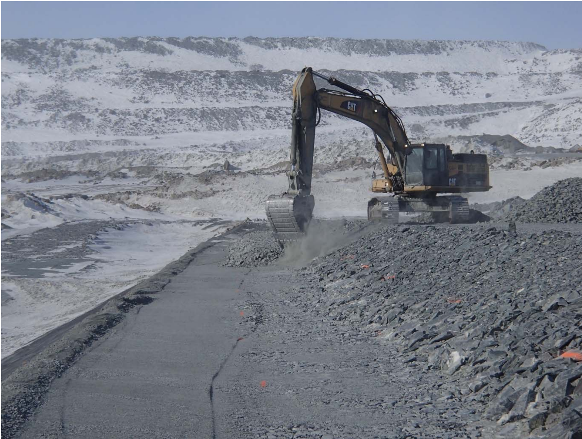
Photograph CD-1832: From Sta. 0+280/-25 m, looking N. Placement of a second 0.5 m thick lift of coarse filter from El. 143.5 m to 144 m with an excavator from Sta. 0+175 m to 0+280 m.
