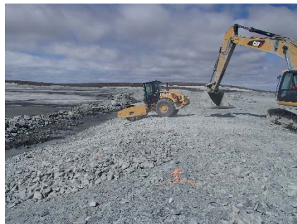
NCIS-035 (2018-06-21), looking N from Sta. 2+550/-25 m. Compaction of the 0.5 m lift (approx.) of coarse filter between El. 150 and 152 m with a 10-tonne smooth-drum compactor (4 passes) in the upstream slope from Sta. 2+524 m to 2+450 m.
