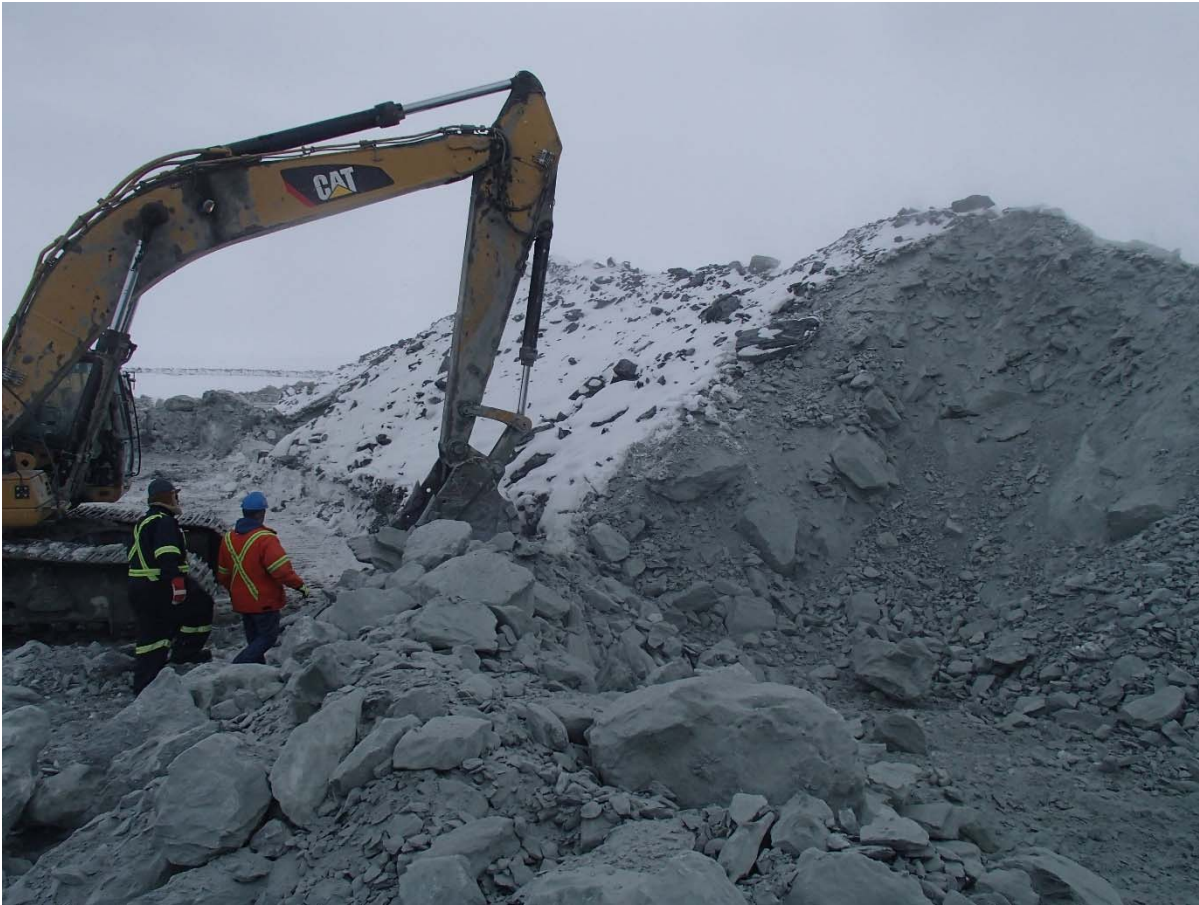
Photograph NCIS-003: Excavation of the snow-rich upstream toe material on an average width of 2 to 3 m with an excavator.
