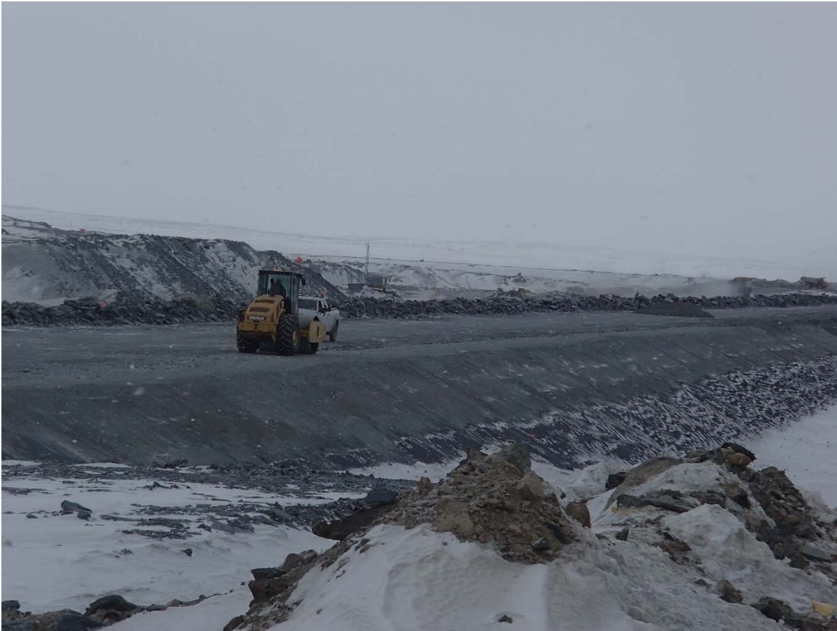
Photograph CD-1847: From Sta. 0+085/-48 m, looking SE. Compaction of the fourth 0.5 m lift (approx.) of fine and coarse filters material at El. 145 m with a 10-tonne smooth-drum compactor with vibration (4 passes) from Sta. 0+170 m to 40+730 m.
