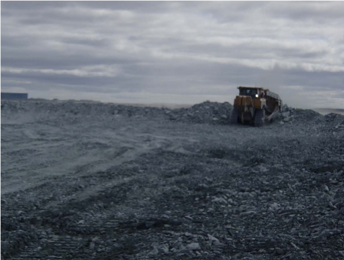
Photograph NCIS-044: From Sta. 1+200/-19 m (approx.), looking S. Placement of a 1.5 to 2 m thick (approx.) lift of UM rockfill from El. 148 m to El. 150 m (approx.) with a dozer from Sta. 1+150 m to 1+120 m (-92 m to +10 m). The material is of good quality and is well graded.
