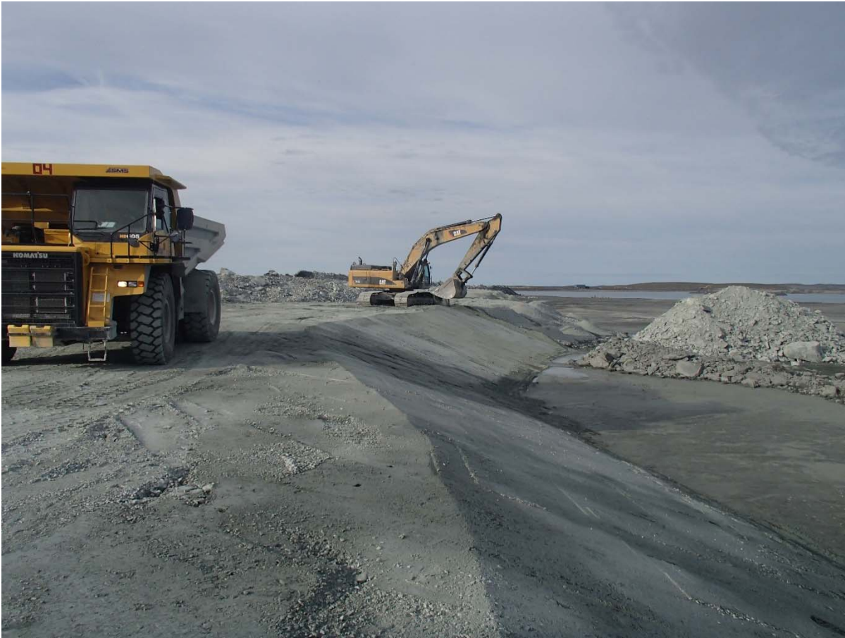
Photograph NCIS-081: From Sta2+975/-37 m (approx.), looking SE. Placement of a 0.5 m thick lift of fine filter over the coarse filter in the upstream slope from El. 150 m to 152 m with an excavator from Sta. 1+300 m to 1+210 m and from Sta. 2+940 m to 3+120 m.
