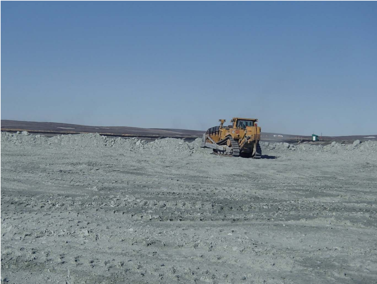
Photograph NCIS-052: From Sta. 1+120/-87 m (approx.), looking SW. Placement of a 1.5 to 2 m thick (approx.) lift of UM rockfill from El. 148 m to El. 150 m (approx.) with a dozer from Sta. 1+115 m to 1+100 m (-107 m to -45 m). The material is of good quality and is well graded.
