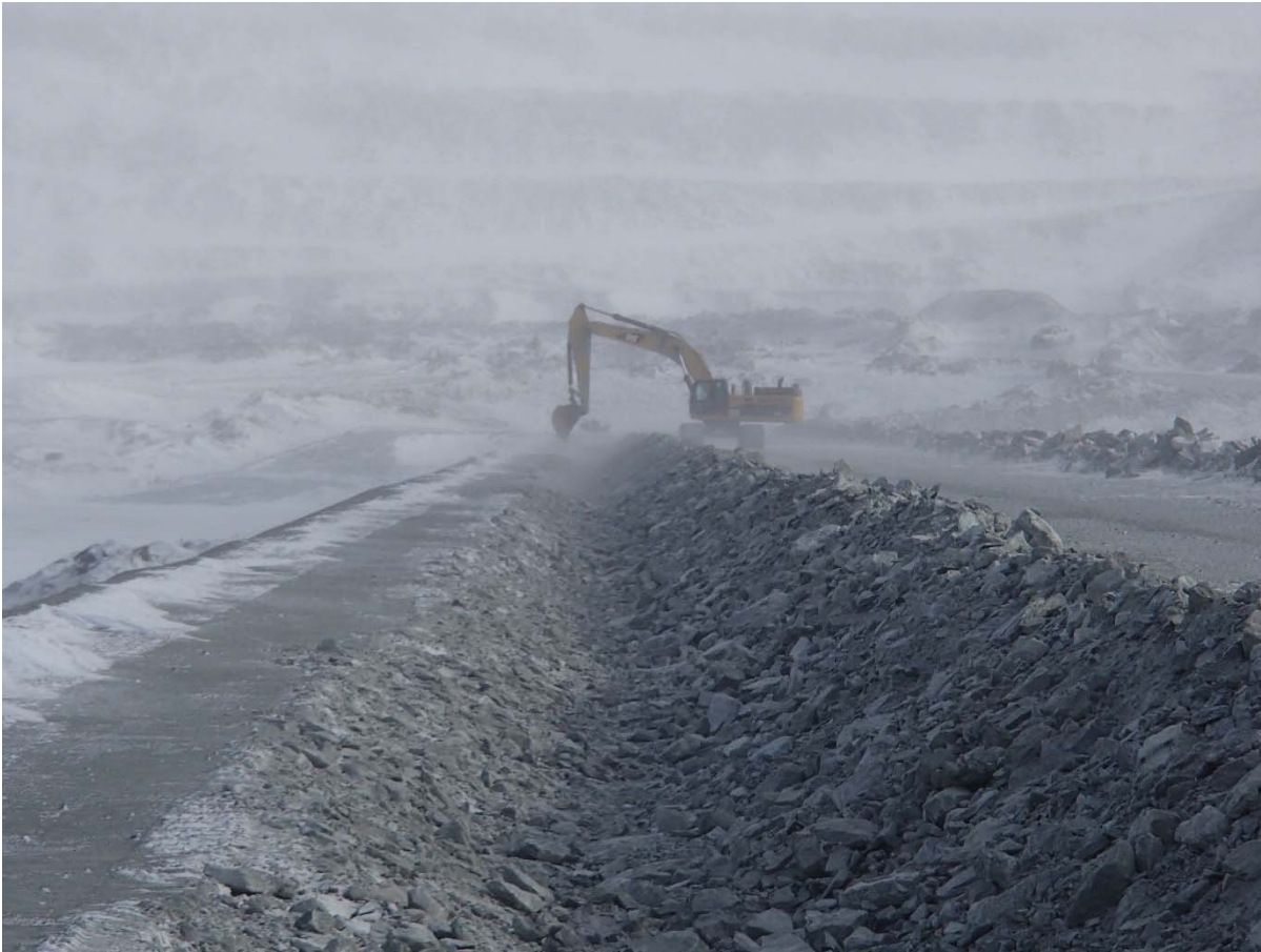
Photograph CD-1852: From Sta. 0+500/-25 m, looking N. Excavation of the LLDPE geomembrane crest anchoring trench from Sta. 0+830 m to 0+170 m.
