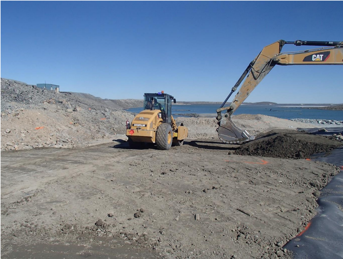
Photograph SD3-339: From Sta. 20+600/-29 m, looking E. Compaction of a first 0.5 m thick lift of compacted sieved till on the upstream toe liner tie-in with an excavator from Sta. 20+588 m to 20+599 m.
