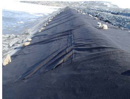
CD-1881 (2018-06-02), looking N from Sta. 0+530/-27 m. View of a geotextile panel with a horizontal weld in the slope at Sta. 0+520 m before its removal.
