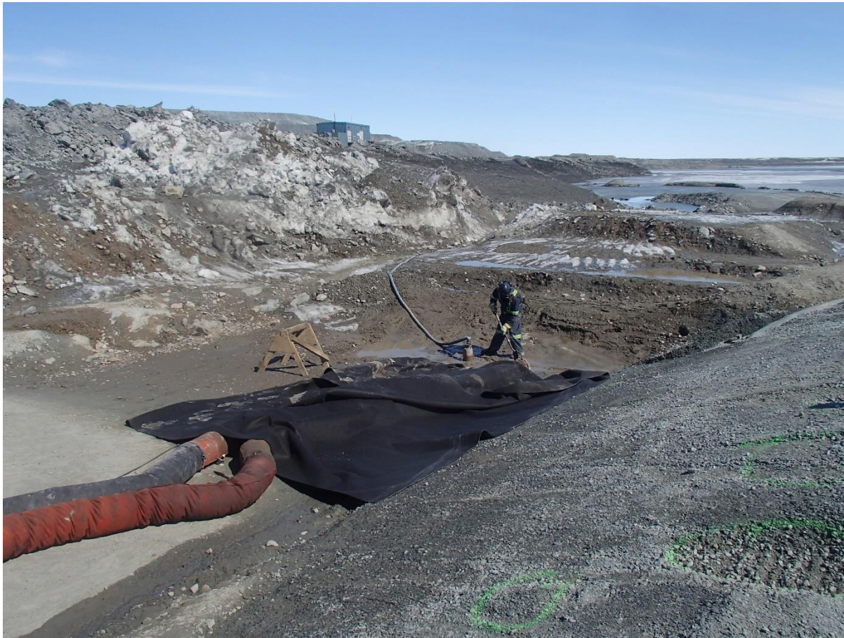
Photograph SD3-305: From Sta. 20+610/-48 m, looking NW. Dewatering of the water ponding on the first compacted sieved till layer of upstream toe liner tie-in. A Genset Frost-fighter is heating the sieved till layer and a pump is evacuating the water.
