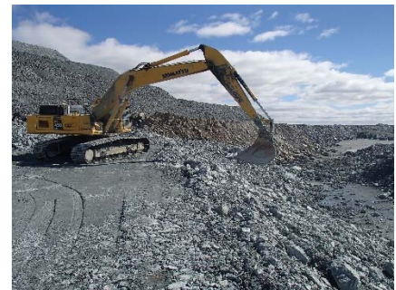
NCIS-045 (2018-06-25), looking S from Sta. 2+760/-40 m. Profiling of the upstream slope (3H:1V) from El. 150 to 152 m with an excavator from Sta. 2+715 m to 2+825 m.
