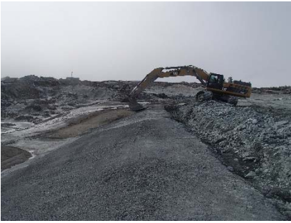
SD3-306 (2018-06-06), looking S from Sta. 20+780/-25 m. Correction of the surface of the fine filter in the upstream slope and the top of the first class compacted sieved till layer with an excavator from Sta. 20+803 m to 20+793 m.
