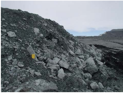
NCIS-028 (2018-06-09), looking E from Sta. 1+340/+3 m. View of the UM rockfill lift approximately 3.2 m thick.
