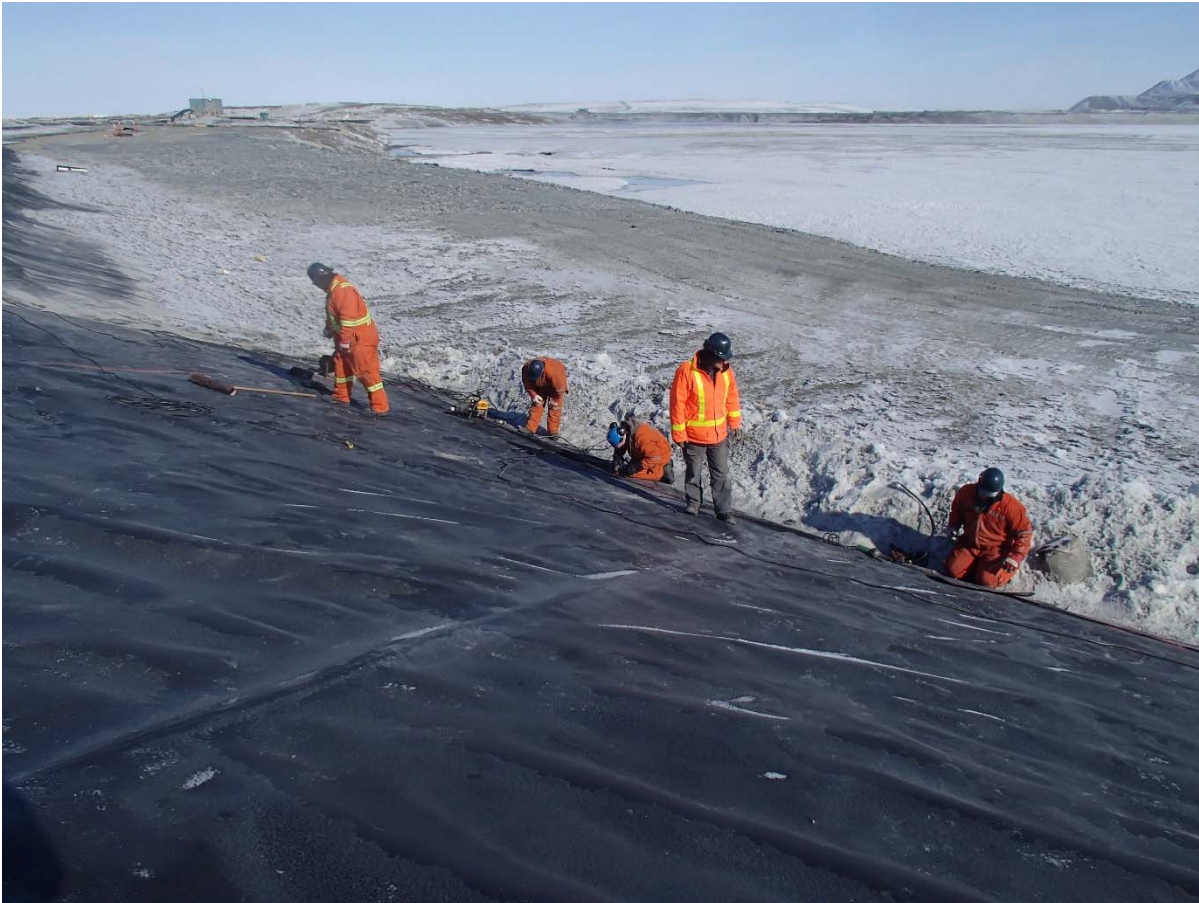
Photograph CD-1865: From Sta. 40+740/-35 m, looking NW. Repairs on the extrusion fillet seam at the bottom of the LLDPE liner panels between Sta. 40+680 m and 0+950 m, on panels 802 to 807, and 811 to 813.
