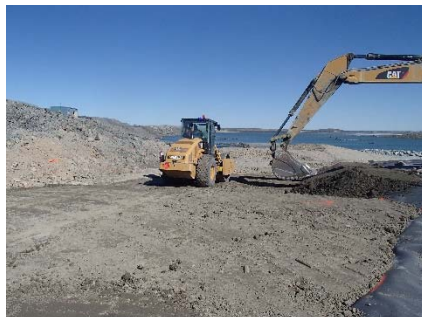
SD3-339 (2018-07-15), looking E from Sta. 20+600/-29 m. Compaction of a first 0.5 m thick lift of compacted sieved till on the upstream toe liner tie-in with an excavator from Sta. 20+588 m to 20+599 m.
