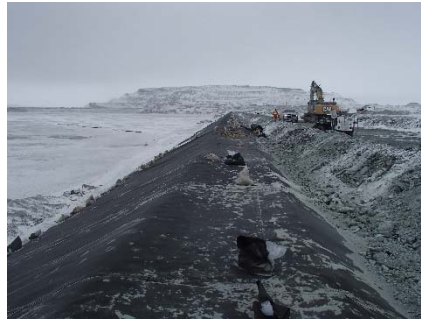
CD-1860 (2018-05-23), looking N from Sta. 0+790/-26 m. Installation of the geotextile on the upstream slope 2H:1V between El. 143 m and 145 m from Sta. 0+830 m to 0+750 m.
