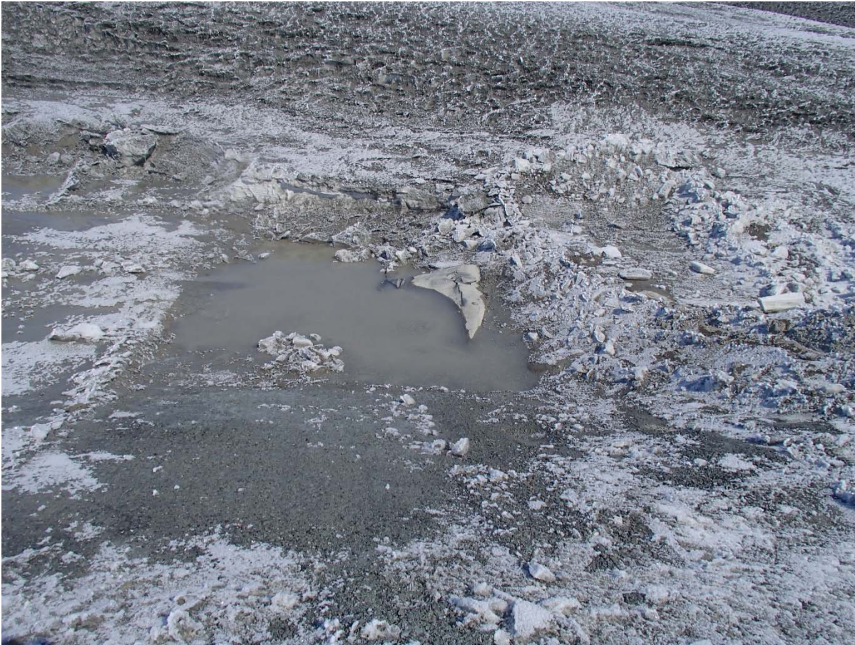
Photograph SD3-302: From Sta. 20+595/42 m, looking NE. View of water ponding on the first compacted sieved till layer of upstream toe liner tie-in. A portion of exposed damaged LLDPE liner is visible.
