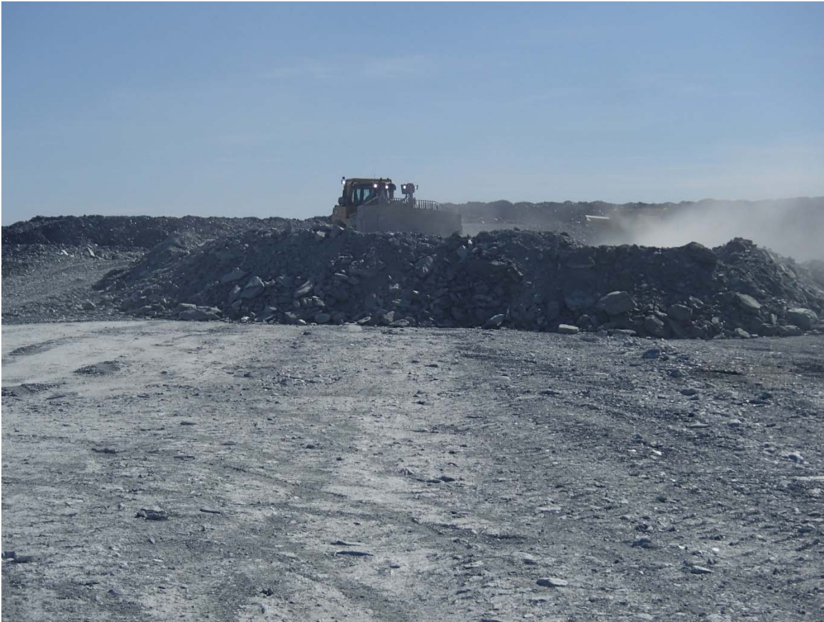
Photograph NCIS-098: From Sta. 2+040/-9 m (approx.), looking E. Placement of a 2 m thick (approx.) lift of UM rockfill from El. 152 m to El. 154 m (approx.) with a dozer from Sta. 2+103 m to 1+984 m (+7 m to -22 m). The material is of good quality and is well graded.
