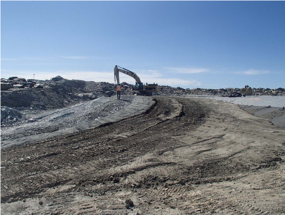
Photograph SD3-336: From Sta. 20+755/-48 m, looking S. Placement of a fourth 0.5 m thick lifts of fine filter, coarse filter and fine rockfill on the upstream slope of the upstream toe liner tie-in with an excavator from Sta. 20+770 to 20+800 m.
