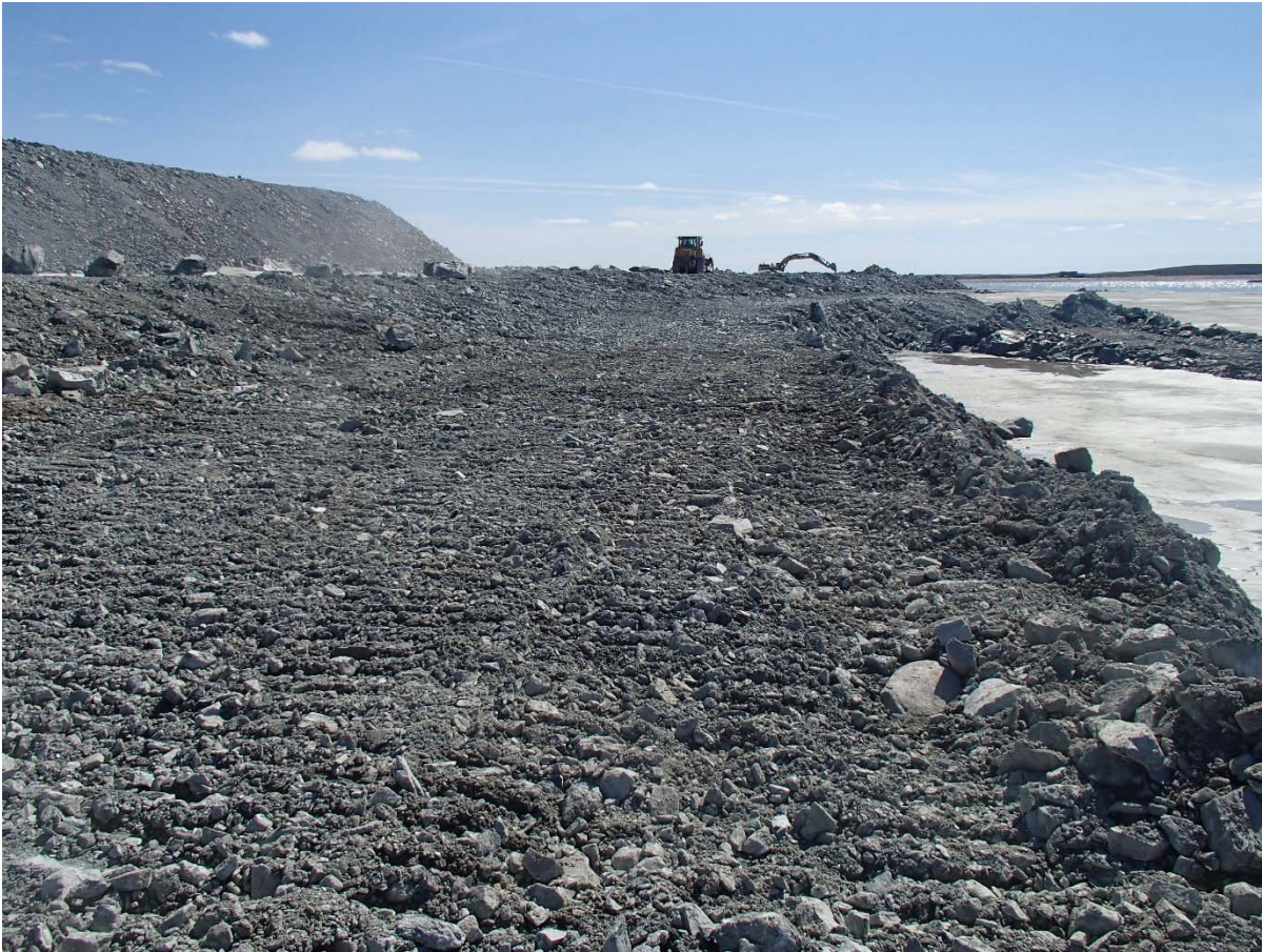
Photograph NCIS-053: From Sta. 2+840/-37 m (approx.), looking S. Removing of UM rockfill material from the capping with a dozer to level the surface to El. 152 m from Sta. 2+850 m to 2+980 m (offset -38 to -24 m).
