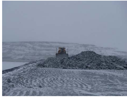
CD-1806 (2018-04-28), looking N from Sta. 0+800/-27 m. Placement a 2 m thick (approx.) lift of intermediate volcanic (IV) rockfill from El. 143 m to El. 145 m from approx. Sta. 0+710 to 0+760m (o.s. -28 to 3 m).
