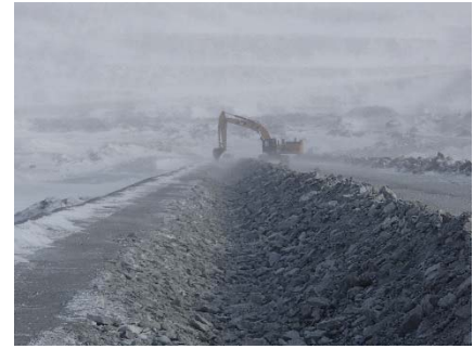
CD-1852 (2018-05-14), looking N from Sta. 0+500/-25 m. Excavation of the LLDPE geomembrane crest anchoring trench from Sta. 0+830 m to 0+170 m.
