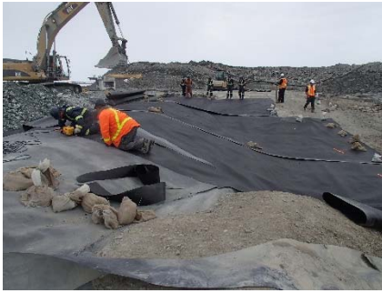
SD3-315 (2018-06-08), looking W from Sta. 20+615/-46 m. Installation of the geotextile on the upstream slope 3H:1V between El. 143 m and 145 m from Sta. 20+593 m to 20+610 m and installation of the LLDPE liner on the upstream slope 3H:1V between El. 143 m and 145 m from Sta. 20+593 m to 20+610 m (panel numbers 965 to 967).
