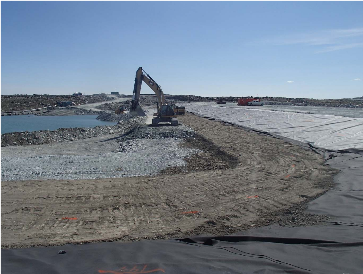
Photograph SD3-330: From Sta. 20+610/-43 m, looking S. Placement of a second 0.5 m thick lift of fine rockfill (0-500 mm) upstream of the low quality till (0-150 mm) from El. 142.5 m to 143 m from Sta. 20+610 m to 20+760 m.
