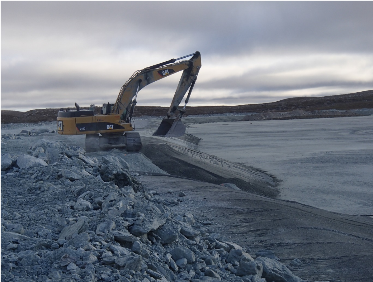
Photograph NCIS-073: From Sta. 1+300/-33 m (approx.), looking N. Placement of a 0.5 m thick lift of fine filter over the coarse filter in the upstream slope from El. 150 m to 152 m with an excavator from Sta. 1+320 m to 1+300 m.
