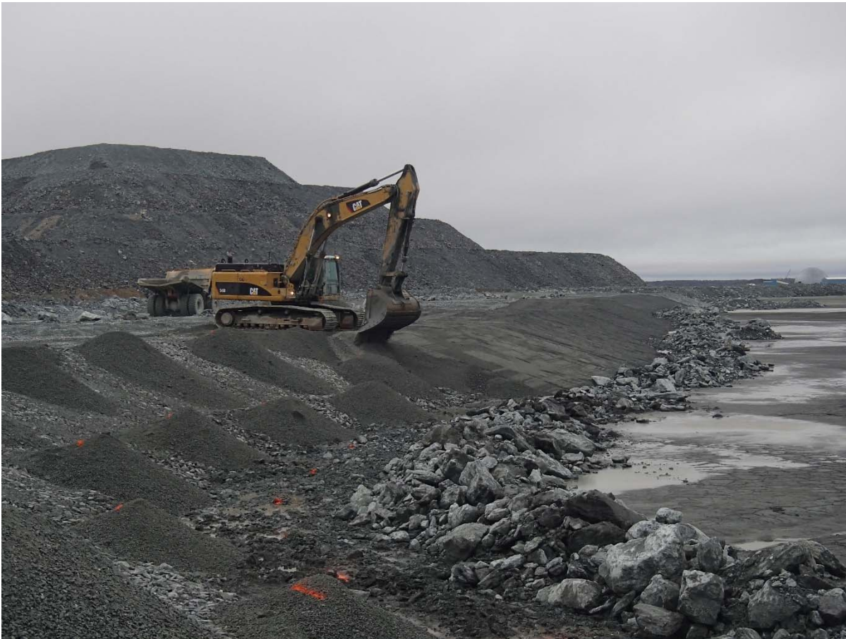
Photograph NCIS-042: From Sta. 2+210/-27 m (approx.), looking SE. Placement of a 0.5 m thick lift of fine filter over the coarse filter in the upstream slope from El. 150 m to 152 m with an excavator from Sta. 2+305 m to 2+040 m.
