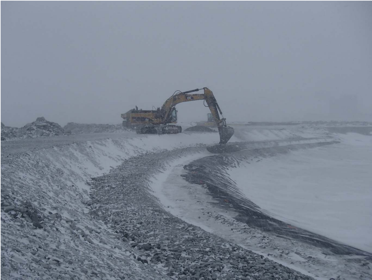
Photograph CD-1827: From Sta 0+940/-16 m, looking SW. Placement of a 0.5 m thick lift of fine filter from El. 143 m to 143.5 m with an excavator from Sta. 40+730 m to 0+ 835 m.
