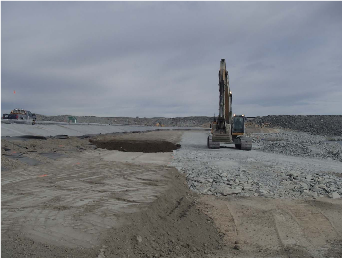
Photograph SD3-345: From Sta. 20+760/-42 m, looking NW. Placement of a fourth 0.5 m thick lift of low quality till (0-150 mm) from El. 143 m to 143.5 m from Sta. 20+619 m to 20+777 m.
