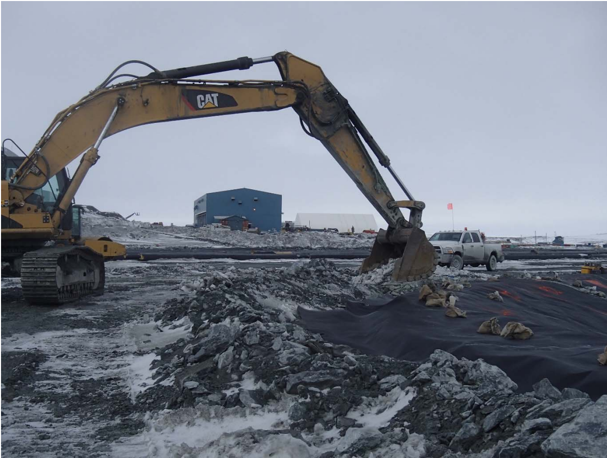
Photograph CD-1863: From Sta. 40+750/-18 m, looking SW. Backfilling of the geosynthetics tie-in from Sta. 40+680 m to 0+950 m.
