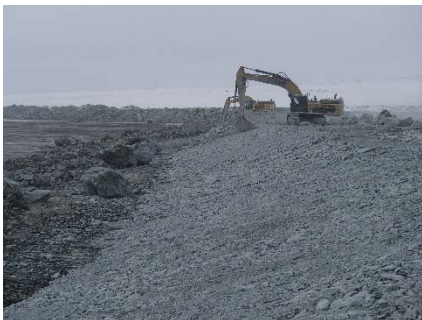
NCIS-007 (2018-05-20). Profiling of the upstream slope (3H:1V) from El. 150 to 152 m with an excavator.
