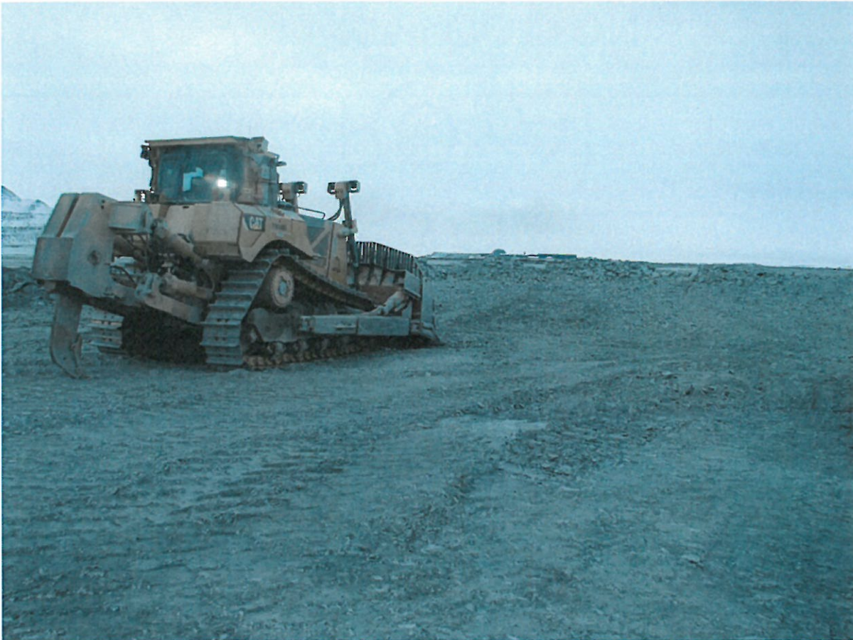
Photograph NCIS-020: From Sta. 1+570 m (approx.), looking S. Placement of a 2 m thick (approx.) lift of UM rockfill from El. 150 m to El. 152 m (approx.) with a dozer from Sta. 1+564 m to 1+535 m (offset unavailable).
