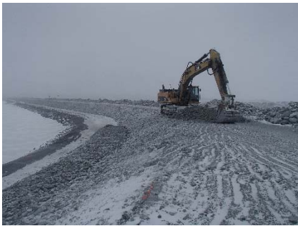
CD-1826 (2018-05-06), looking NE from Sta. 40+770/-27 m. Placement of a 0.5 m thick lift of coarse filter from El. 143 m to 143.5 m with an excavator from Sta. 40+730 m to 0+775 m.
