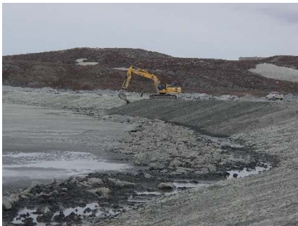
NCIS-040 (2018-06-24), looking W from Sta. 2+185/-25 m. Placement of a 0.5 m thick lift of fine filter over the coarse filter in the upstream slope from El. 150 m to 152 m with an excavator from Sta. 2+305 m to 2+460 m and from Sta. 1+980 m to 1+835 m.
