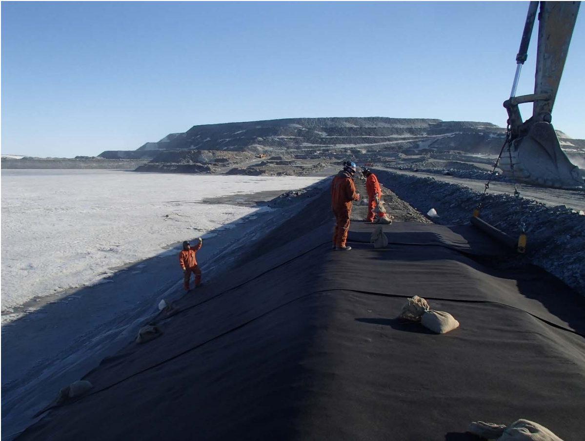
Photograph CD-1885: From Sta. 0+460/-26 m, looking N. Installation of the geotextile on the upstream slope 2H:1V between El. 143 m and 145 m from Sta. 0+480 m to 0+320 m.
