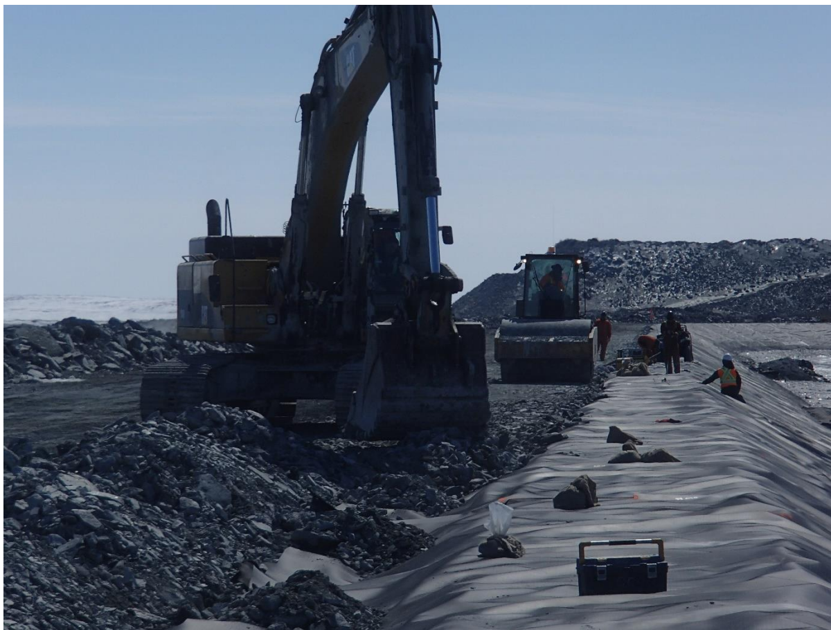
Photograph CD-1884: From Sta. 0+530/-25 m, looking S. Backfilling of the geosynthetics tie-in from Sta. 0+610 m to 0+480 m and compaction of the tie-in material with a 10-tonne smooth-drum compactor with vibration (4 passes) from Sta.0+610 to 0+480 m.
