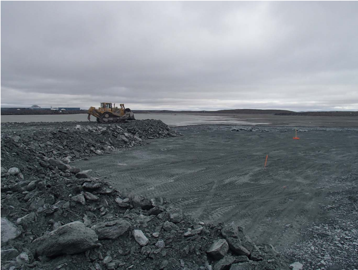
Photograph NCIS-083: From Sta 1+140/-52 m (approx.), looking SW. Placement of a 2 m thick (approx.) lift of IV rockfill from El. 150 m to El. 152 m (approx.) with a dozer from Sta. 1+160 m to 1+170 m (-64 m to -111 m). The material is of good quality and is well graded.
