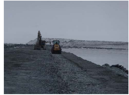
CD-1843 (2018-05-10), looking S from Sta. 0+460/-23 m. Compaction of the third 0.5 m lift (approx.) of fine and coarse filters material at El. 144.5 m with a 10-tonne smooth-drum compactor with vibration (4 passes) from Sta 0+335m to 0+900 m.
