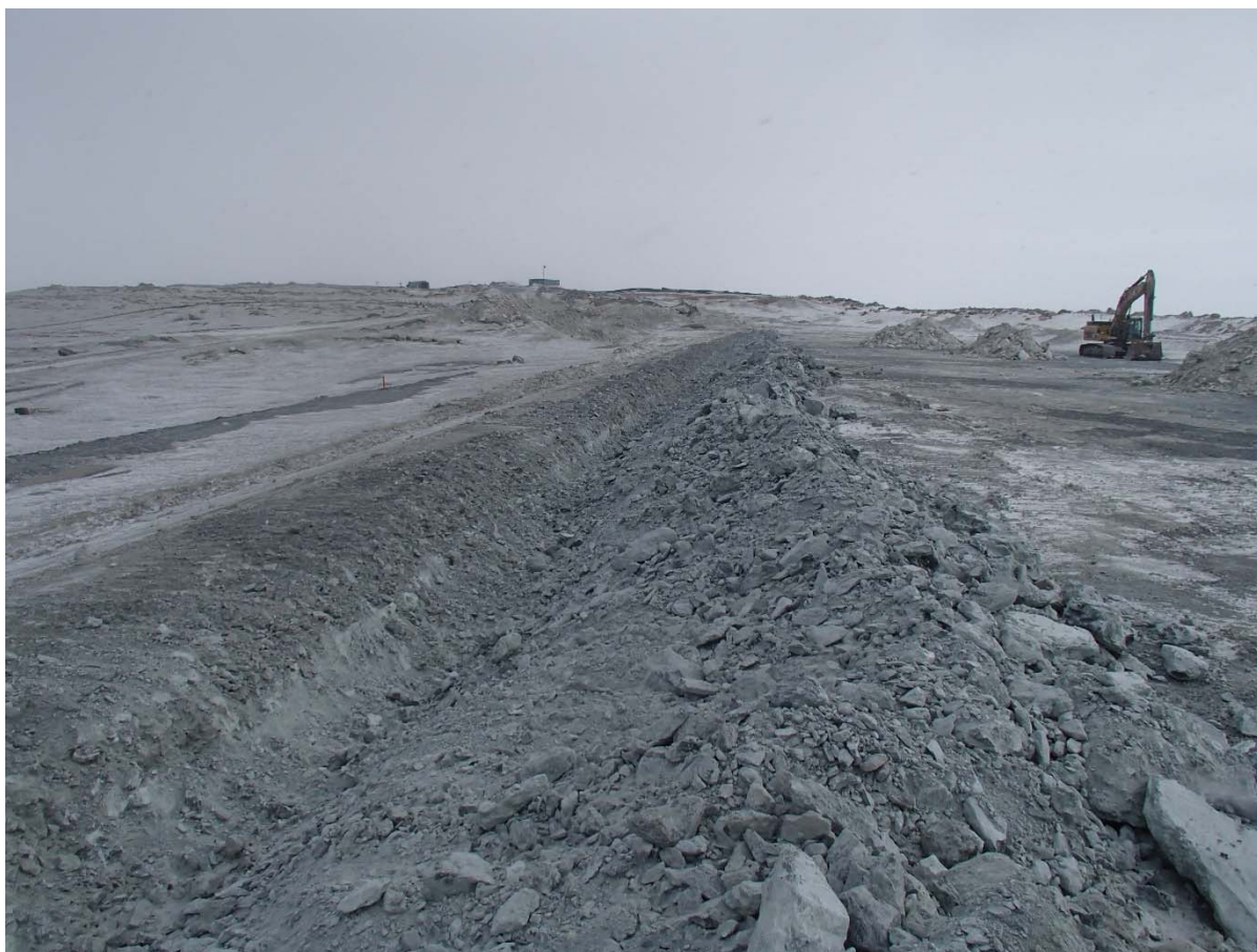
Photograph SD3-301: From Sta. 20+660/-22 m, looking SE. Excavation of the LLDPE geomembrane crest anchoring trench with an excavator from Sta. 20+655 m to 20+675 m.
