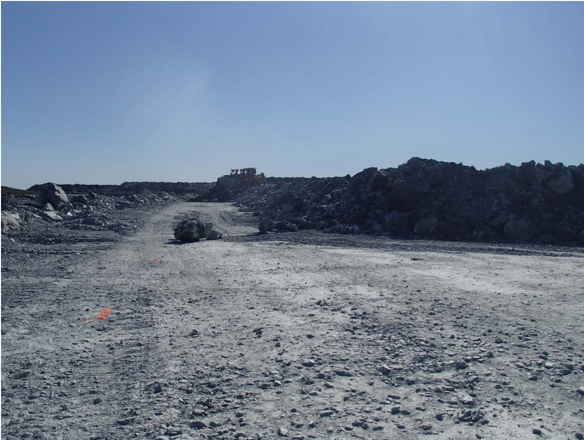
Photograph NCIS-100: From Sta. 1+960/+10 m (approx.), looking E. Placement of a 2 m thick (approx.) lift of UM rockfill from El. 152 m to El. 154 m (approx.) with a dozer from Sta. 1+984 m to 1+947 m (+14 m to -26 m). The material is of good quality and is well graded.
