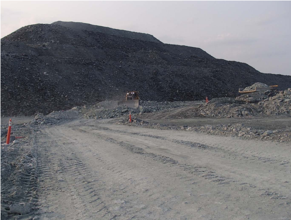
Photograph NCIS-086: From Sta 2+750/+14 m (approx.), looking E. Placement of a 2 m thick (approx.) lift of UM rockfill from El. 152 m to El. 154 m (approx.) with a dozer from Sta. 2+780 m to 2+760 m (-60 m to -44 m).
