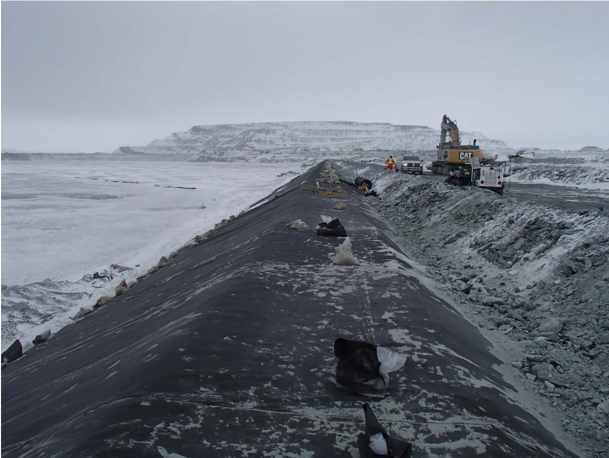
Photograph CD-1860: From Sta. 0+790/-26 m, looking N. Installation of the geotextile on the upstream slope 2H:1V between El. 143 m and 145 m from Sta. 0+830 m to 0+750 m.
