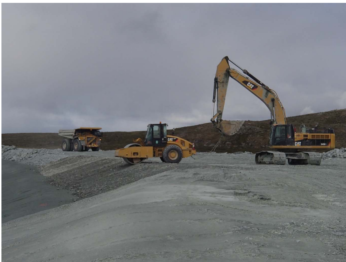
Photograph NCIS-131: From Sta. 1+940/-20 m (approx.), looking W. Compaction of the 0.5 m lift (approx.) of coarse filter between El. 152 m and 154 m with a 10-tonne smooth-drum compactor with vibration (4 passes) in the upstream slope from Sta. 1+890 m to 1+826 m.
