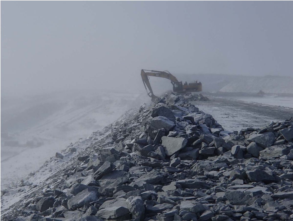
Photograph CD-1825: From Sta 0+430/+9 m, looking S. Profiling of the downstream slope (1.5H:1V) from El. 143 to 145 m with an excavator between Sta. 0+330 m and 0+440 m and between Sta. 0+530 m and 0+745 m.
