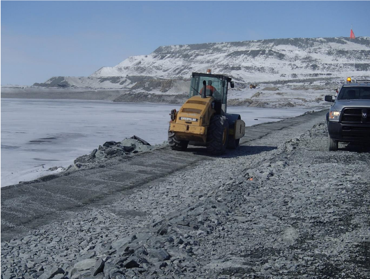
Photograph CD-1840: From Sta 0+575/-15 m, looking NW. Compaction of the second 0.5 m lift (approx.) of fine and coarse filters material at El. 144 m with a 10-tonne smooth-drum compactor with vibration (4 passes) from Sta 0+500 m to 40+730 m.
