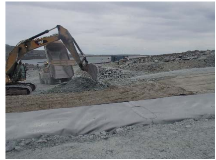
SD3-346 (2018-07-17), looking E from Sta. 20+760/-21 m. Placement of a third 0.5 m thick lift of fine UM rockfill (0-500 mm) upstream of the low quality till (0-150mm) from El. 143 m to 143.5 m from Sta. 20+668 m to 20+777 m.
