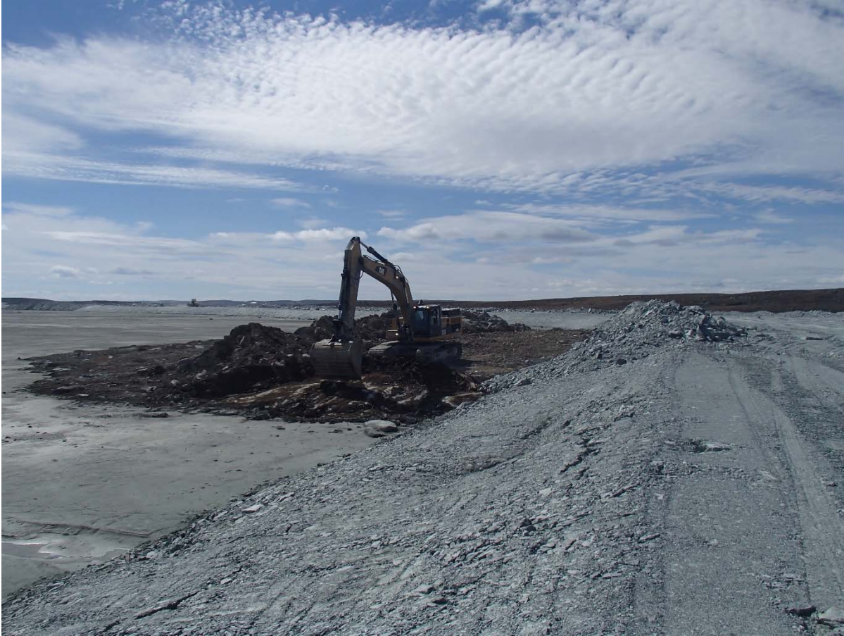
Photograph NCIS-031: From Sta. 1+880/-21 m (approx.), looking SW. Final clean-up of the dike footprint with an excavator to reach a good quality bedrock from Sta. 1+800 to 1+850 m (offset -42 to -33 m).
