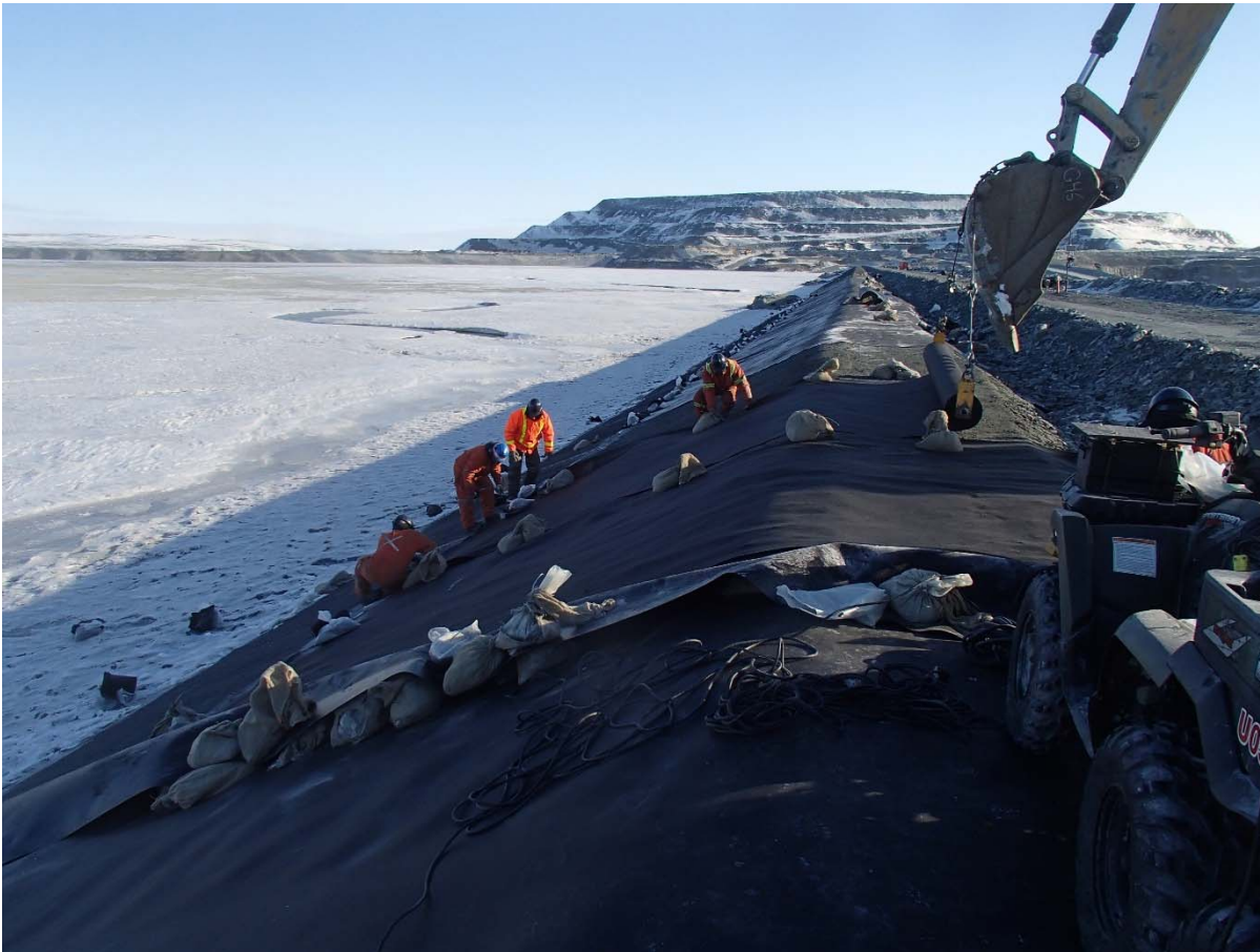
Photograph CD-1871: From Sta. 0+910/-25 m, looking N. Installation of the geotextile on the upstream slope 2H:1V between El. 143 m and 145 m from Sta. 0+900 m to 0+870 m.
