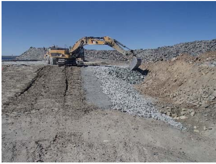
SD3-341 (2018-07-15), looking W from Sta. 20+600/-59 m. Placement of a first 0.5 m thick lift of fine rockfill on the upstream slope of the upstream toe liner tie-in with an excavator from Sta. 20+588 m to 20+599 m.
