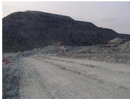
NCIS-086 (2018-07-10), looking E from Sta. 2+750/+14 m (approx.). Placement of a 2 m thick (approx.) lift of UM rockfill from El. 152 m to El. 154 m (approx.) with a dozer from Sta. 2+780 m to 2+760 m (-60 m to -44 m).
