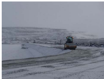
CD-1848 (2018-05-13), looking N from Sta. 40+780/-15 m. Compaction of the fourth 0.5 m lift (approx.) of fine and coarse filters material at El. 145 m with a 10-tonne smooth-drum compactor with vibration (4 passes) from Sta 0+930 m to 40+730 m.
