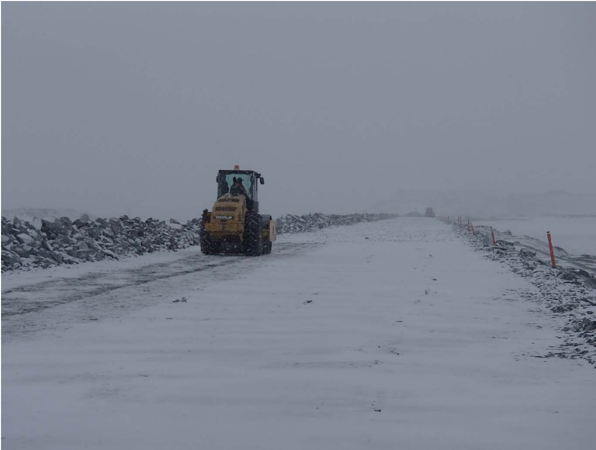
Photograph CD-1807: From Sta. 0+200/-15 m looking S. Compaction of the 2 m lift (approx.) of IV rockfill at El. 145 m with a 10-tonne smooth-drum compactor with vibration (6 passes) from Sta. 0+150 to 0+280 m (o.s. -21 to 11 m).
