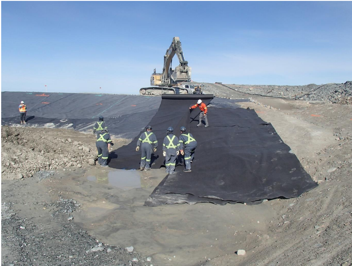
Photograph SD3-322: From Sta. 20+625/-63 m, looking W. Installation of two layers of geotextile on the upstream slope 3H:1V between El. 142 m and 143 m (approx.) from Sta. 20+610 m to 20+800 m.
