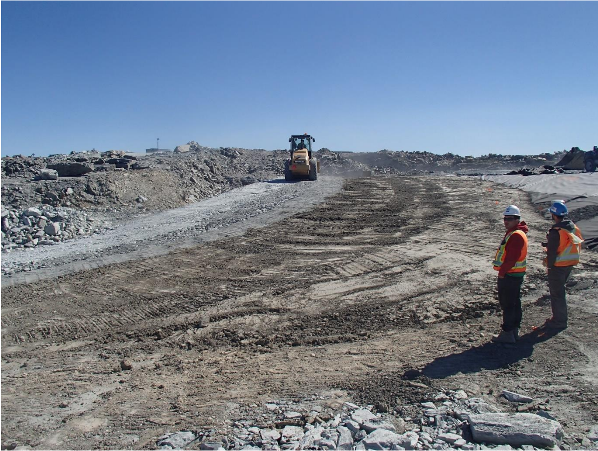
Photograph SD3-337: From Sta. 20+760/-37 m, looking S. Compaction of the fourth 0.5 m thick lifts of fine filter, coarse filter and fine rockfill on the upstream slope of the upstream toe liner tie-in with a 10 tonne smooth-drum compactor with vibrations (4 passes) from Sta. 20+770 to 20+800 m.
