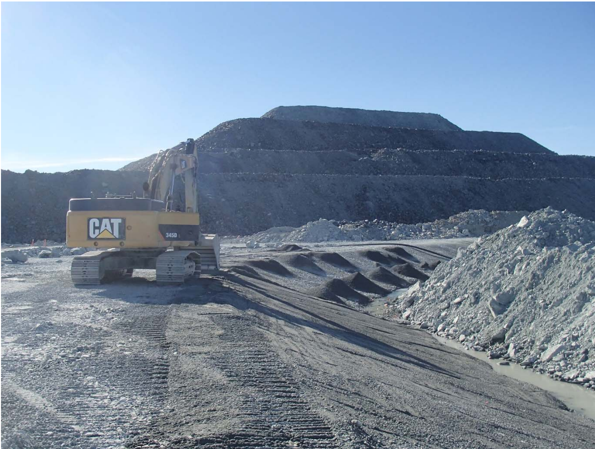
Photograph NCIS-071: From Sta. 2+670/-28 m (approx.), looking SE. Placement of a 0.5 m thick lift of fine filter over the coarse filter in the upstream slope from El. 150 m to 152 m with an excavator from Sta. 1+550 m to 1+320 m and 1+630 m to 1+610 m.
