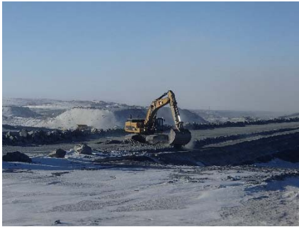
CD-1844 (2018-05-11), looking SE from Sta. 0+080/-49 m. Placement of a fourth 0.5 m thick lift of coarse filter from El. 144.5 m to 145 m with an excavator from Sta. 0+170 m to 40+730 m.
