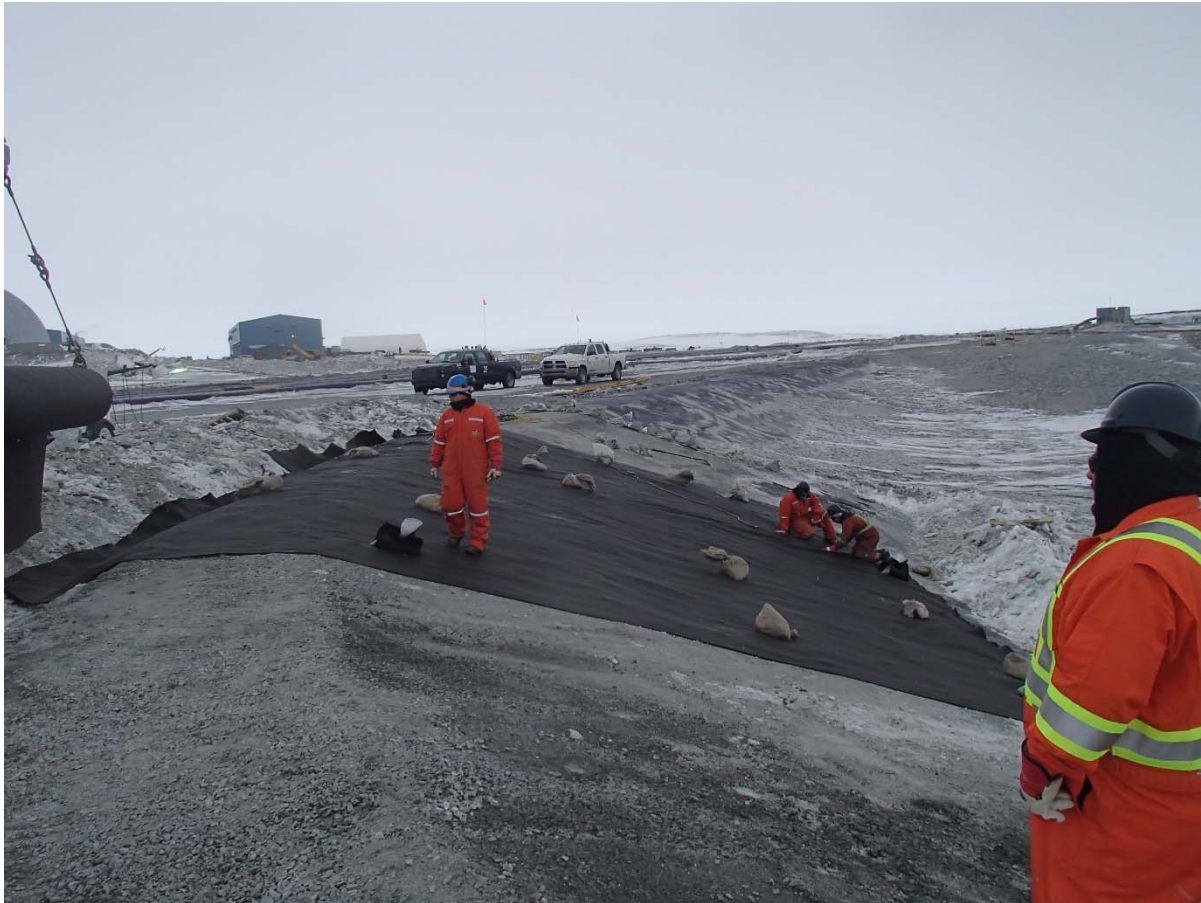
Photograph CD-1859: From Sta. 40+780/-38 m, looking SW. Installation of the geotextile on the upstream slope 3H:1V (SD5 side) to 2H:1V (Central Dike side) between El. 143 m and 145 m from Sta. 40+640 m to 0+830 m.
