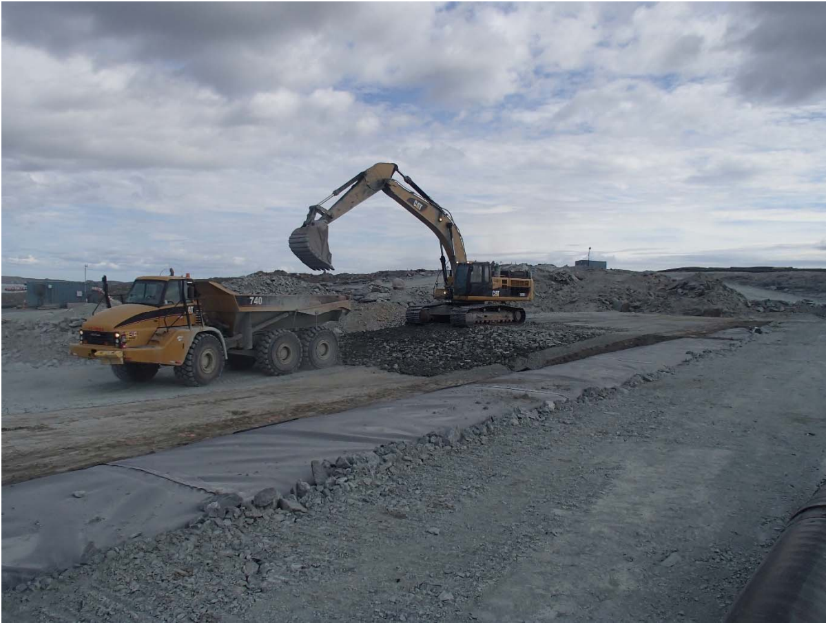
Photograph SD3-350: From Sta. 20+740/-24 m, looking SE. Placement of a 0.5 m thick lift of coarse filter on the top of the fine filter on the upstream toe liner tie-in with an excavator from Sta. 20+777 m to 20+807 m.
