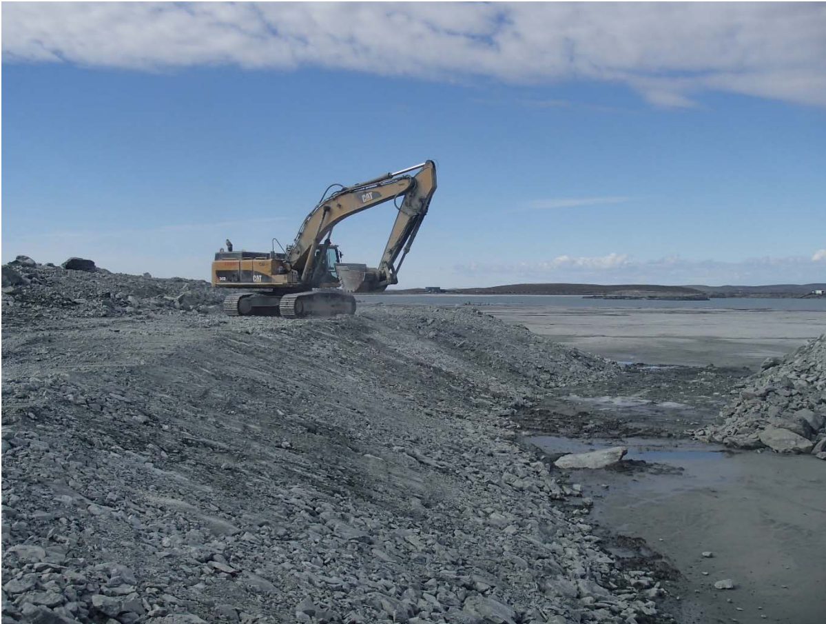
Photograph NCIS-067: From Sta. 2+880/-26 m (approx.), looking SW. Profiling of the upstream slope (3H:1V) from El. 150 to 152 m with an excavator from Sta. 2+860 m to 2+975 m.
