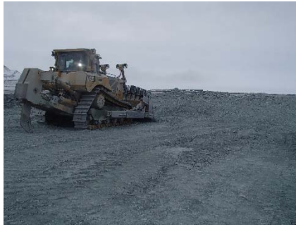
NCIS-020 (2018-05-27), looking S from Sta. 1+570 m. Placement a 2 m thick (approx.) lift of UM rockfill from El. 150 m to El. 152 m (approx.) with a dozer from Sta. 1+564 m to 1+535 m (o.s. unavailable).
