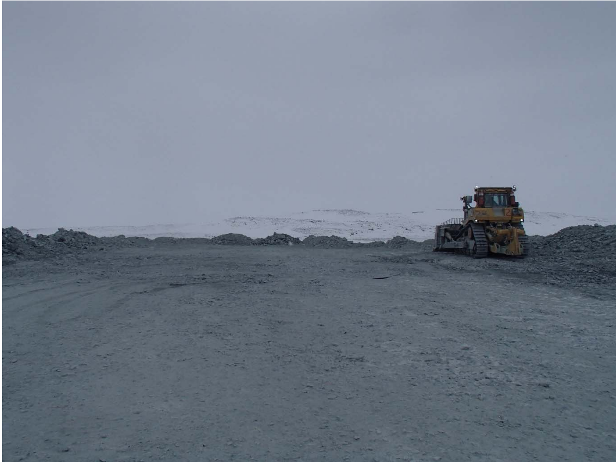
Photograph NCIS-009: Placement of a 2 m thick (approx.) lift of UM rockfill from El. 150 m to El. 152 m (approx.) with a dozer from Sta. 1+880 m to 1+825 m (offset unavailable).
