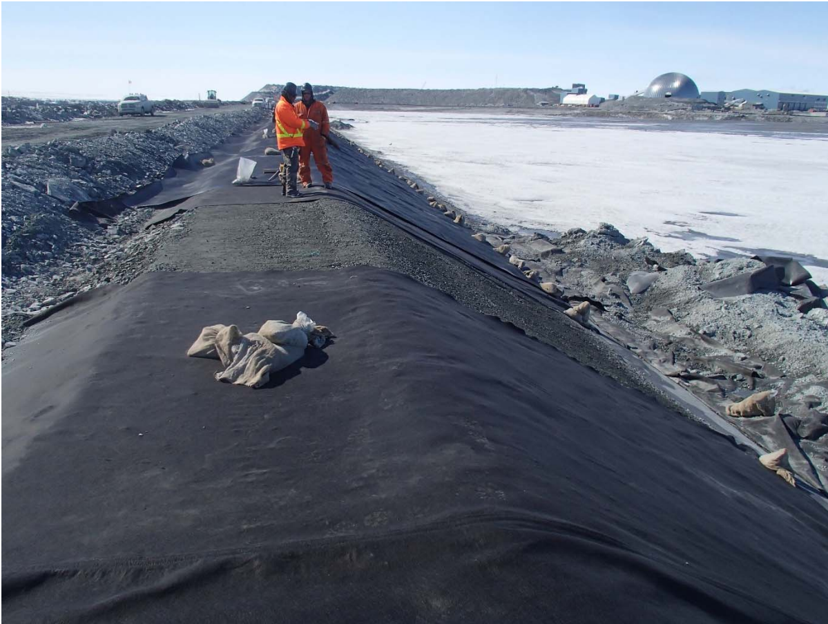
Photograph CD-1882: From Sta. 0+510/-25 m, looking S. View of the emplacement of the geotextile panel with a horizontal weld in the slope at Sta. 0+520 following its removal.
