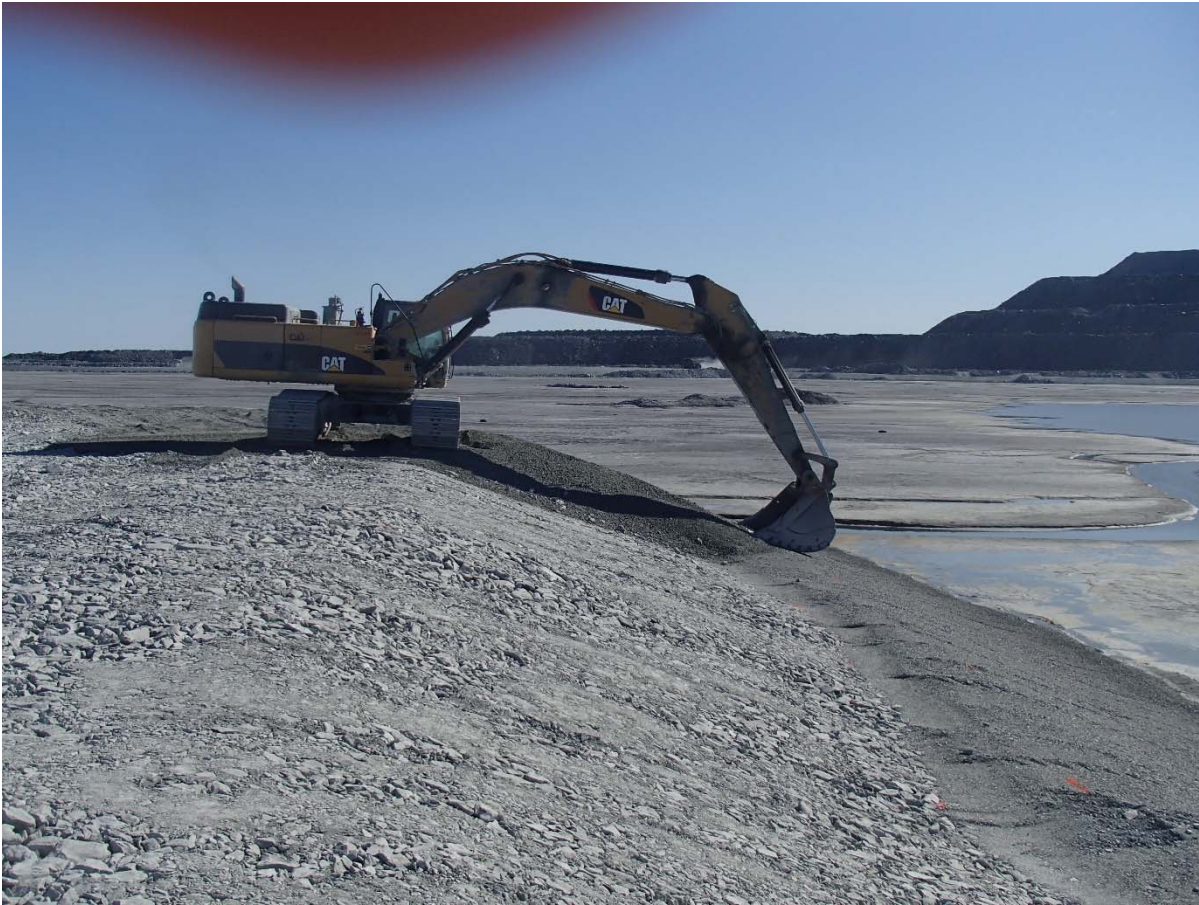
Photograph NCIS-101: From Sta. 1+120/-89 m (approx.), looking N. Placement of a 0.5 m thick lift of fine filter in the upstream slope from El. 150 m to 152 m with an excavator from Sta. 1+113 m to 1+205 m.
