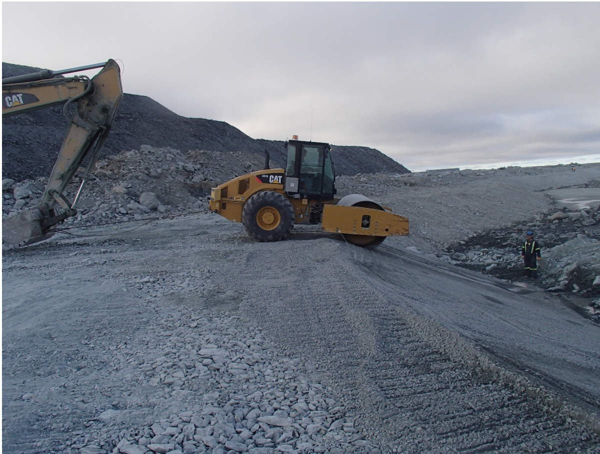
Photograph NCIS-074: From Sta. 2+750/-37 m (approx.), looking SE. Compaction of the 0.5 m lift (approx.) of fine filter between El. 150 and 152 m with a 10-tonne smooth-drum compactor (4 passes) in the upstream slope from Sta. 2+810 m to 2+095 m. Vibration is used except for the first pass down the slope in order to stabilize the material and limit deformation of the lift.
