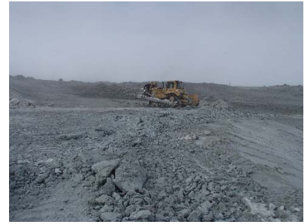
SD3-299 (2018-05-16), looking NW from Sta. 20+620/-26 m. Scarification of the frozen ultramafic volcanic (UM) rockfill on the crest with a dozer for the anchoring trench excavation between Sta. 20+605 m and 20+780 m.
