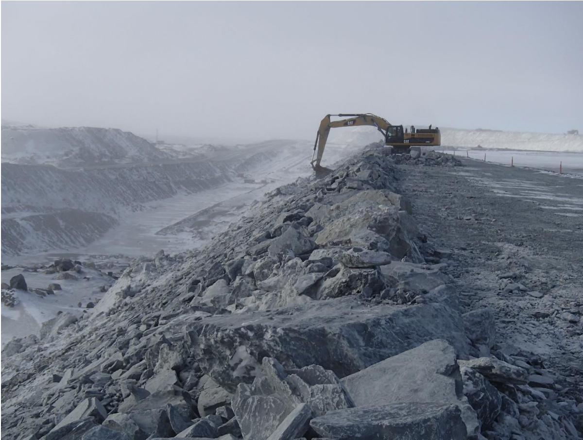
Photograph CD-1821: From Sta. 0+175/+3, looking S. Profiling of the downstream slope (1.5H:1V) from El. 143 to 145 m with an excavator between Sta. 0+250 m and 0+330 m.
