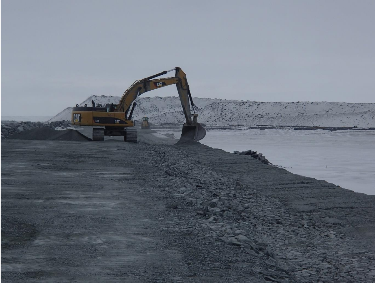
Photograph CD-1842: From Sta 0+380/-16 m, looking S. Placement of a third 0.5 m thick lift of fine filter from El. 143.5 m to 144 m upstream of the coarse filter with an excavator from Sta. 0+335 m to 0+940 m.
