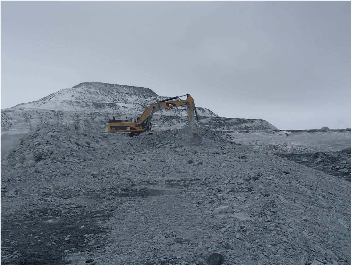
Photograph NCIS-013: From Sta. 2+600 m (approx.), looking NE. Correction of the crest elevation with an excavator to achieve a closer elevation to 152 m around Sta. 2+650 m.
