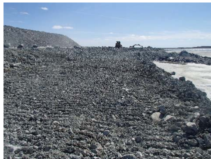
NCIS-053 (2018-06-27), looking S from Sta. 2+840/-37 m. Removing of UM rockfill material from the capping with a dozer to level the surface to El. 152 m from Sta. 2+850 m to 2+980 m (o.s. -38 to -24 m).
