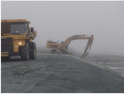
NCIS-082 (2018-07-07), looking S from Sta. 3+060/-33 m. Placement of a 0.5 m thick lift of fine filter over the coarse filter in the upstream slope from El. 150 m to 152 m with an excavator from Sta. 3+120 m to 3+160 m.
