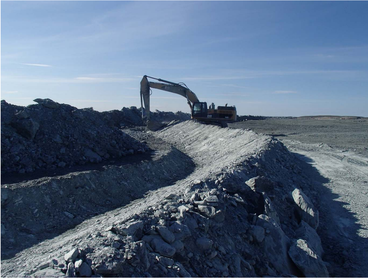
Photograph NCIS-116: From Sta. 1+700/+37 m (approx.), looking SE. Excavation of a 0.8 m (approx.) deep, 1 m wide shallow ditch in the rockfill capping with an excavator from Sta. 1+500 m to 1+455 m.
