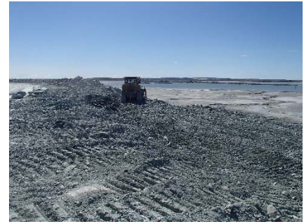
NCIS-057 (2018-06-28), looking SW from Sta. 3+010/-15 m. Removing of UM rockfill material from the capping with a dozer to level the surface to El. 152 m from Sta. 2+980 m to 3+050 m (o.s. -30 to -20 m).
