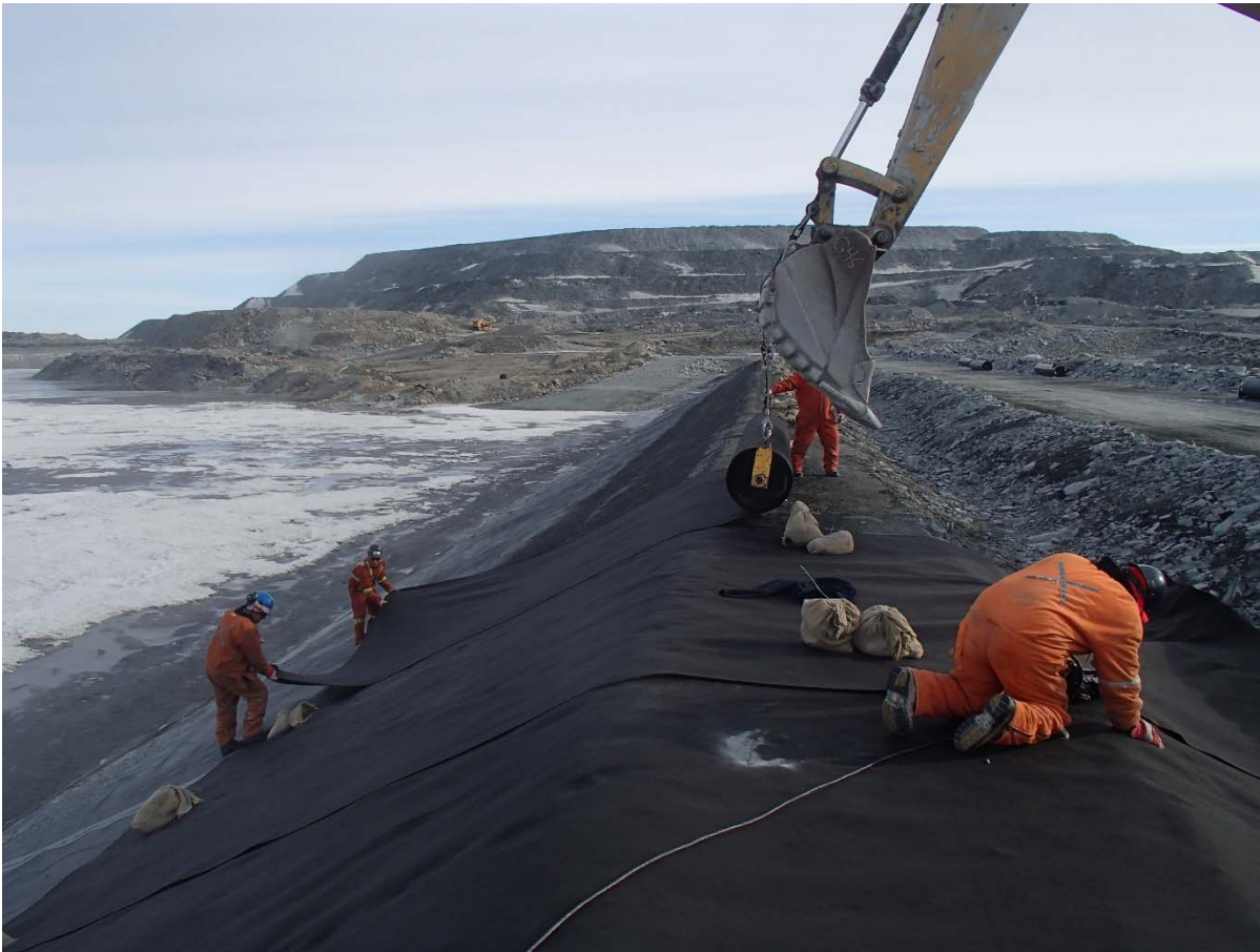
Photograph CD-1887: From Sta. 0+310/-26 m, looking N. Installation of the geotextile on the upstream slope 2H:1V between El. 143 m and 145 m from Sta. 0+320 m to 0+150 m.
