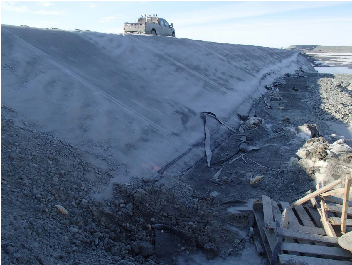
Photograph CD-1892: From Sta. 0+155/-32 m, looking S. View of the liner panel 933 overlapping the underlying liner that has been cut at around Sta. 0+160 m to drain the water.
