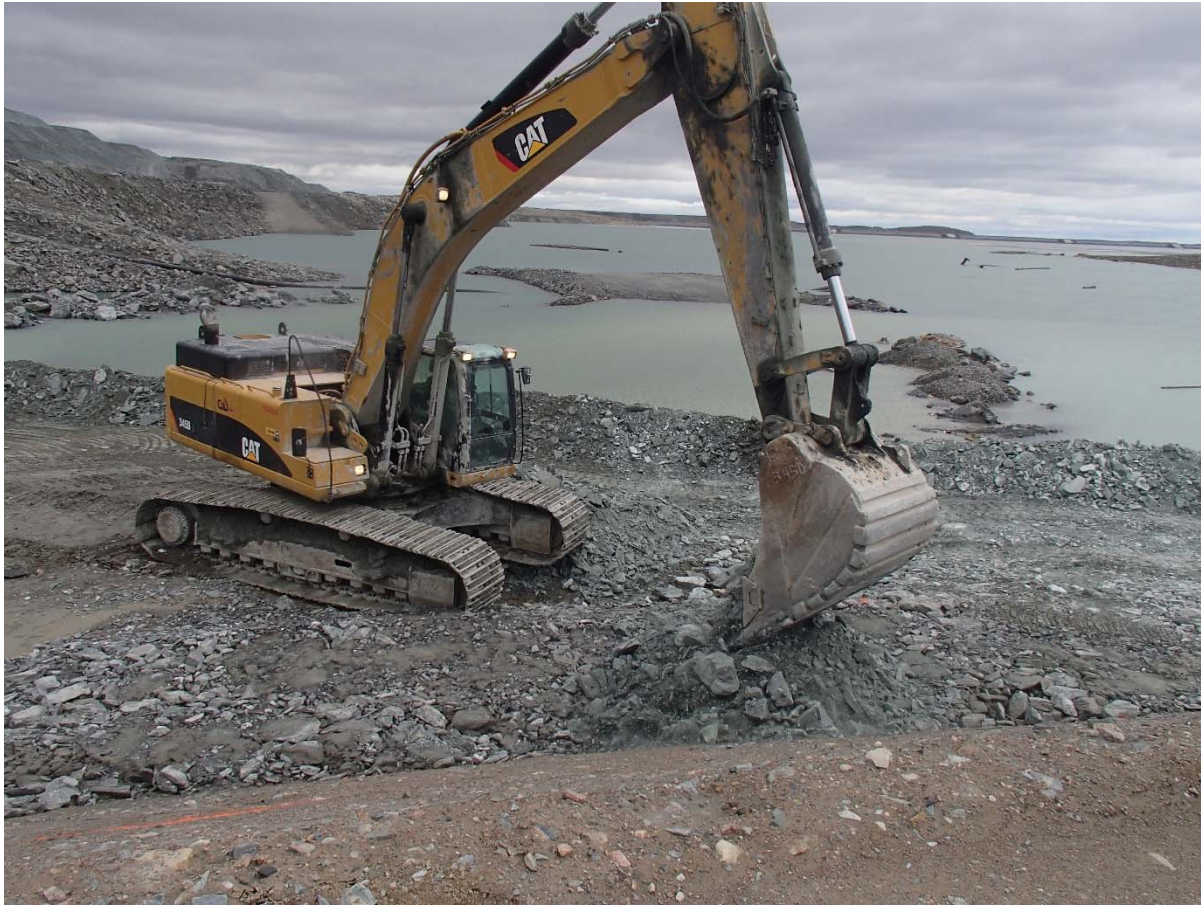
Photograph SD3-320: From Sta. 20+620/-67 m, looking E. Placement of a 1 m thick (approx.) lift of fine IV rockfill over the compacted till in the upstream slope from El. 142 m to 144 m with an excavator from Sta. 20+600 m to 20+610 m.
