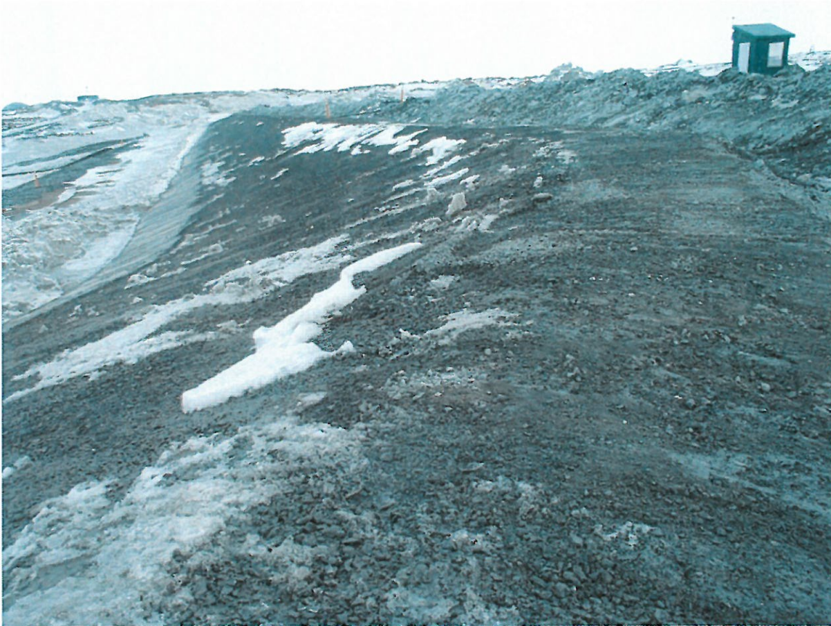
Photograph SD3-304: From Sta. 20+620/-36 m, looking SE. Smoothing of the surface of the fine filter with an excavator on top of the upstream slope from Sta. 20+600 m to 20+780 m.
