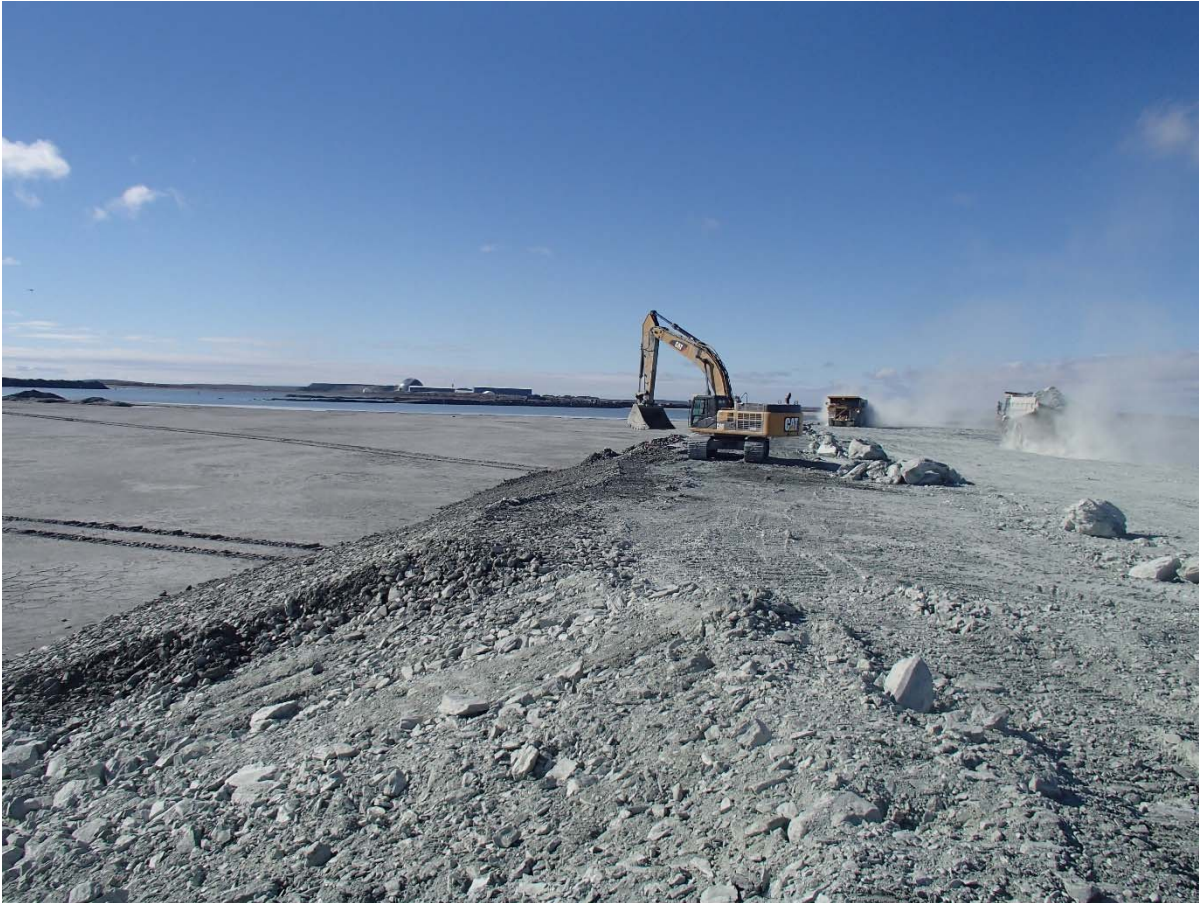
Photograph NCIS-058: From Sta. 1+340/-34 m (approx.), looking S. Placement of a 0.5 m thick lift of coarse filter in the upstream slope from El. 148 m to 152 m with an excavator from Sta. 1+340 m to 1+270 m.
