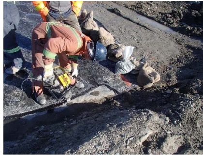
SD3-316 (2018-06-09), looking NW from Sta. 20+610/-45 m. Repairs on the extrusion fillet seam between LLDPE panel 965 and the existing LLDPE panel at Sta. 20+600 m (approx.).
