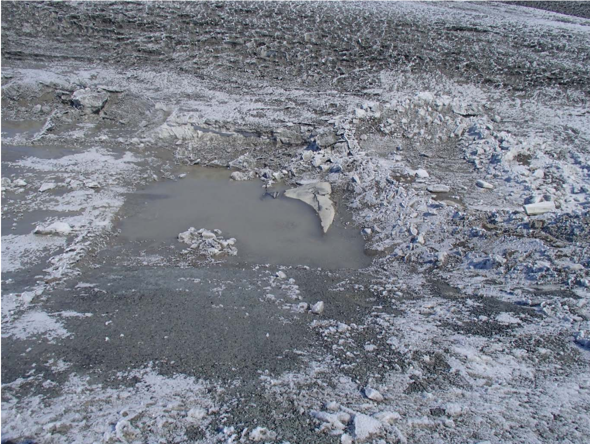
Photograph SD3-302: From Sta. 20+595/42 m, looking NE. View of water ponding on the first compacted sieved till layer of upstream toe liner tie-in. A portion of exposed damaged LLDPE liner is visible.
