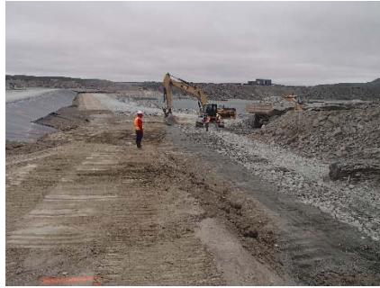
SD3-333 (2018-07-13), looking N from Sta. 20+817/-29 m. Placement of a second 0.5 m thick lift of fine rockfill on the upstream slope of the upstream toe liner tie-in with an excavator from Sta. 20+775 m to 20+800 m.
