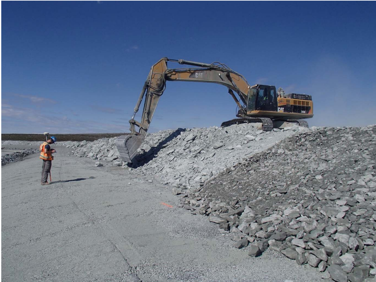
Photograph NCIS-103: From Sta. 2+420/-27 m (approx.), looking NE. Profiling of the upstream slope (3H:1V) from El. 152 to 154 m with an excavator from Sta. 2+400 m to 2+410 m. Oversize boulders were removed.
