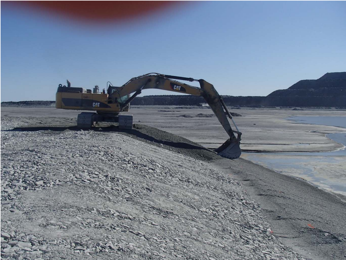
Photograph NCIS-101: From Sta. 1+120/-89 m (approx.), looking N. Placement of a 0.5 m thick lift of fine filter in the upstream slope from El. 150 m to 152 m with an excavator from Sta. 1+113 m to 1+205 m.
