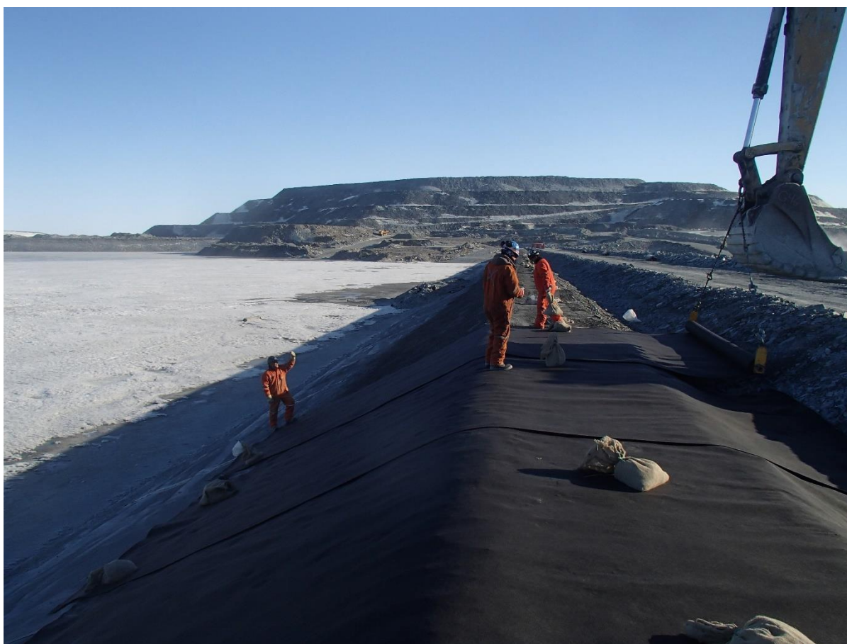
Photograph CD-1885: From Sta. 0+460/-26 m, looking N. Installation of the geotextile on the upstream slope 2H:1V between El. 143 m and 145 m from Sta. 0+480 m to 0+320 m.
