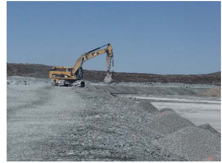
NCIS-066 (2018-06-30), looking N from Sta. 1+400/-34 m. Placement of a 0.5 m thick lift of fine filter over the coarse filter in the upstream slope from El. 150 m to 152 m with an excavator from Sta. 1+595 m to 1+550 m.
