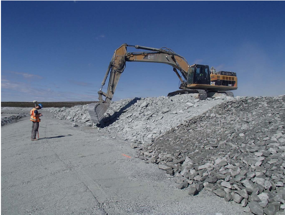
Photograph NCIS-103: From Sta. 2+420/-27 m (approx.), looking NE. Profiling of the upstream slope (3H:1V) from El. 152 to 154 m with an excavator from Sta. 2+400 m to 2+410 m. Oversize boulders were removed.
