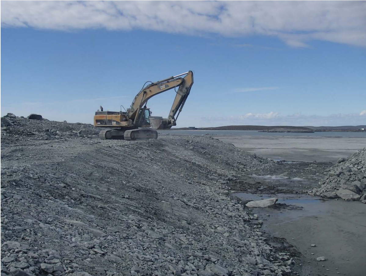
Photograph NCIS-067: From Sta. 2+880/-26 m (approx.), looking SW. Profiling of the upstream slope (3H:1V) from El. 150 to 152 m with an excavator from Sta. 2+860 m to 2+975 m.
