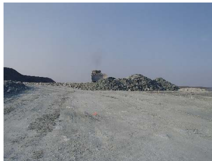
NCIS-089 (2018-07-12), looking S from Sta. 2+525/+4 m (approx.). Placement of a 2 m thick (approx.) lift of UM rockfill from El. 152 m to El. 154 m (approx.) with a dozer from Sta. 2+605 m to 2+455 m (+3 m to -23 m).
