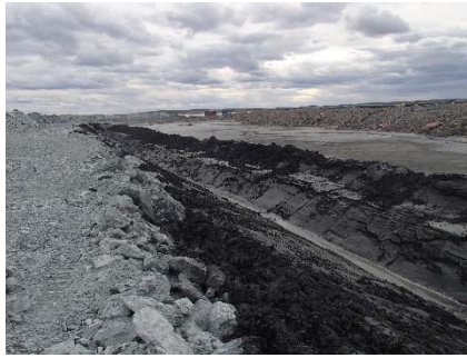
NCIS-137 (2018-07-31), looking SW from Sta. 1+380/+14 m (approx.). Excavation of a 0.8 m (approx.) deep, 1 m wide shallow ditch in the tailings with an excavator from Sta. 1+300 m to 1+200 m.
