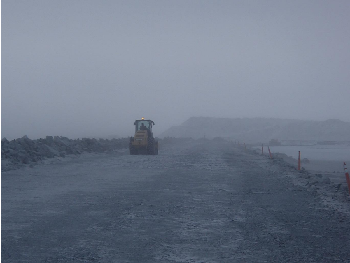
Photograph CD-1810: From Sta. 0+335/-15 m looking S. Compaction of the 2 m lift (approx.) of IV rockfill at El. 145 m with a 10-tonne smooth-drum compactor with vibration (6 passes) from Sta. 0+350 to 0+540 m (o.s. -19 to -7 m).
