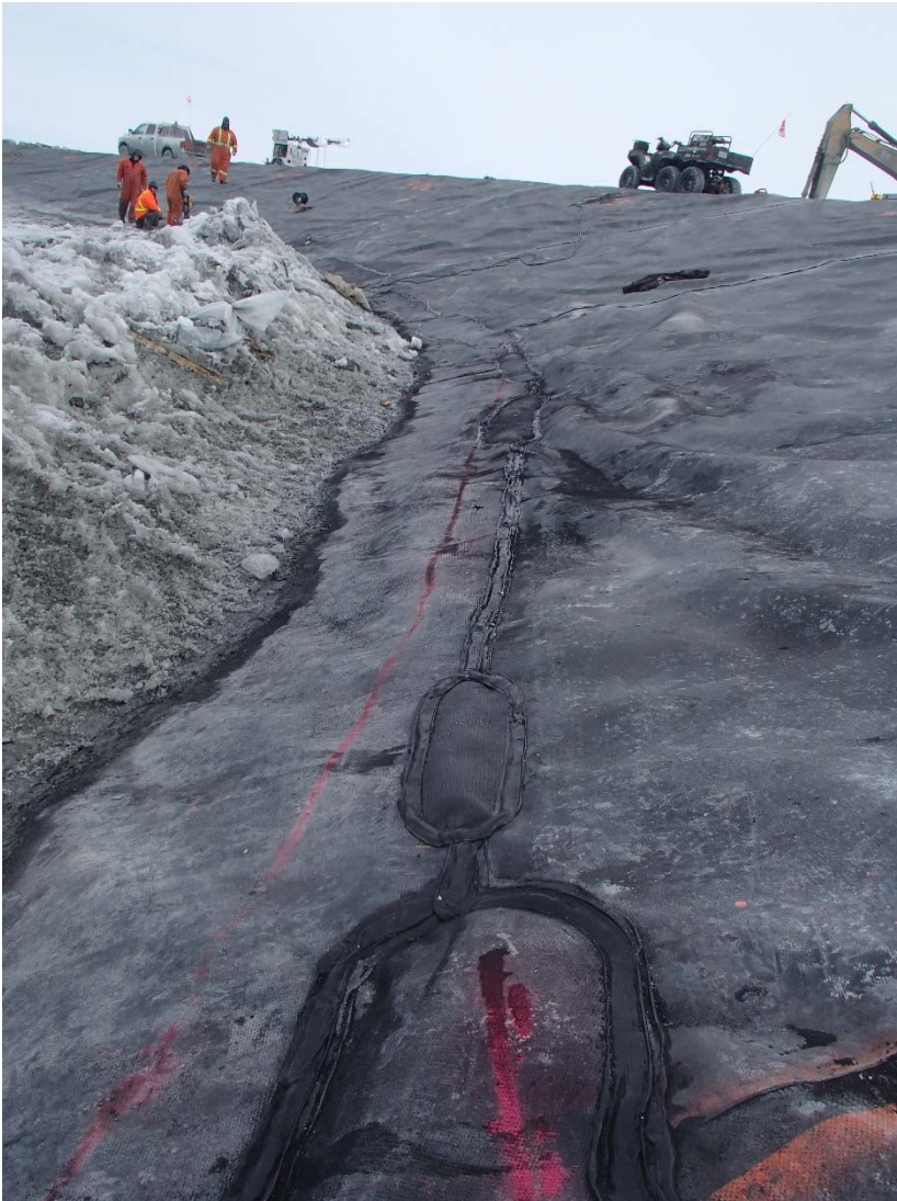
Photograph CD-1867: From Sta. 40+680/-37 m, looking E. View of repair patches on the extrusion weld at the bottom of the panels.
