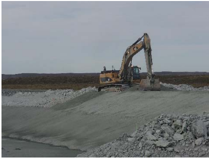
NCIS-136 (2018-07-31), looking SW from Sta. 1+800/-33 m (approx.). Placement of a 0.5 m thick lift of fine filter in the upstream slope from El. 152 m to 154 m with an excavator from Sta. 1+700 m to 1+660 m.
