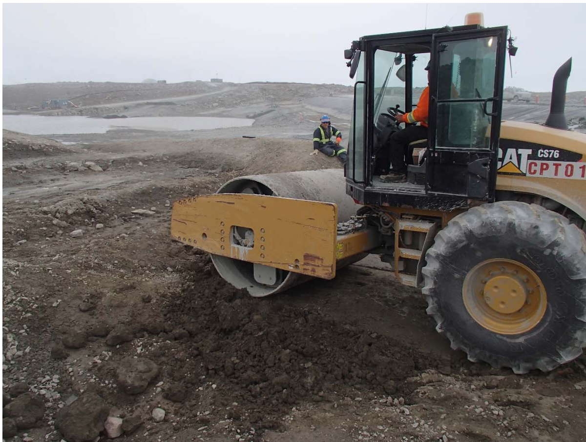
Photograph SD3-313: From Sta. 20+600/-52 m, looking S. Compaction of the 0.15 m-thick lift of compacted sieved till with a 10-tonne smooth-drum compactor without vibration (4 passes) from Sta. 20+596 m to 20+601 m.
