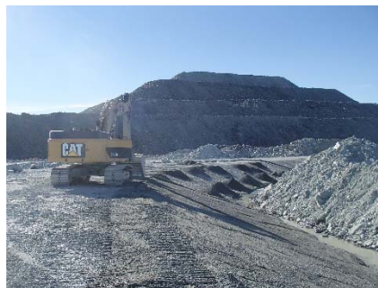
NCIS-071 (2018-07-02), looking SE from Sta. 2+670/-28 m. Placement of a 0.5 m thick lift of fine filter over the coarse filter in the upstream slope from El. 150 m to 152 m with an excavator from Sta. 1+550 m to 1+320 m and 1+630 m to 1+610 m.
