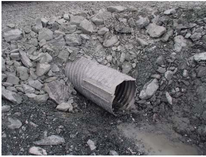
NCIS-127 (2018-07-28), looking SW from Sta. 1+470/+20 m (approx.). View of the culvert installed in the ditch at Sta. 1+460 m.
