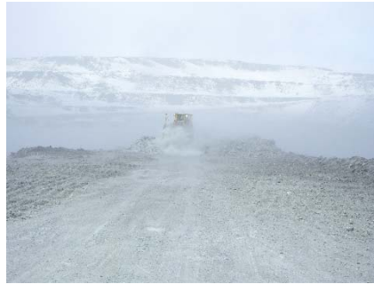
CD-1800 (2018-04-25), looking N from Sta. 0+500/-14 m. Placement a 2 m thick (approx.) lift of intermediate volcanic (IV) rockfill from El. 143 m to El. 145 m from 0+435 to 0+535m (o.s. -28 to -18 m).
