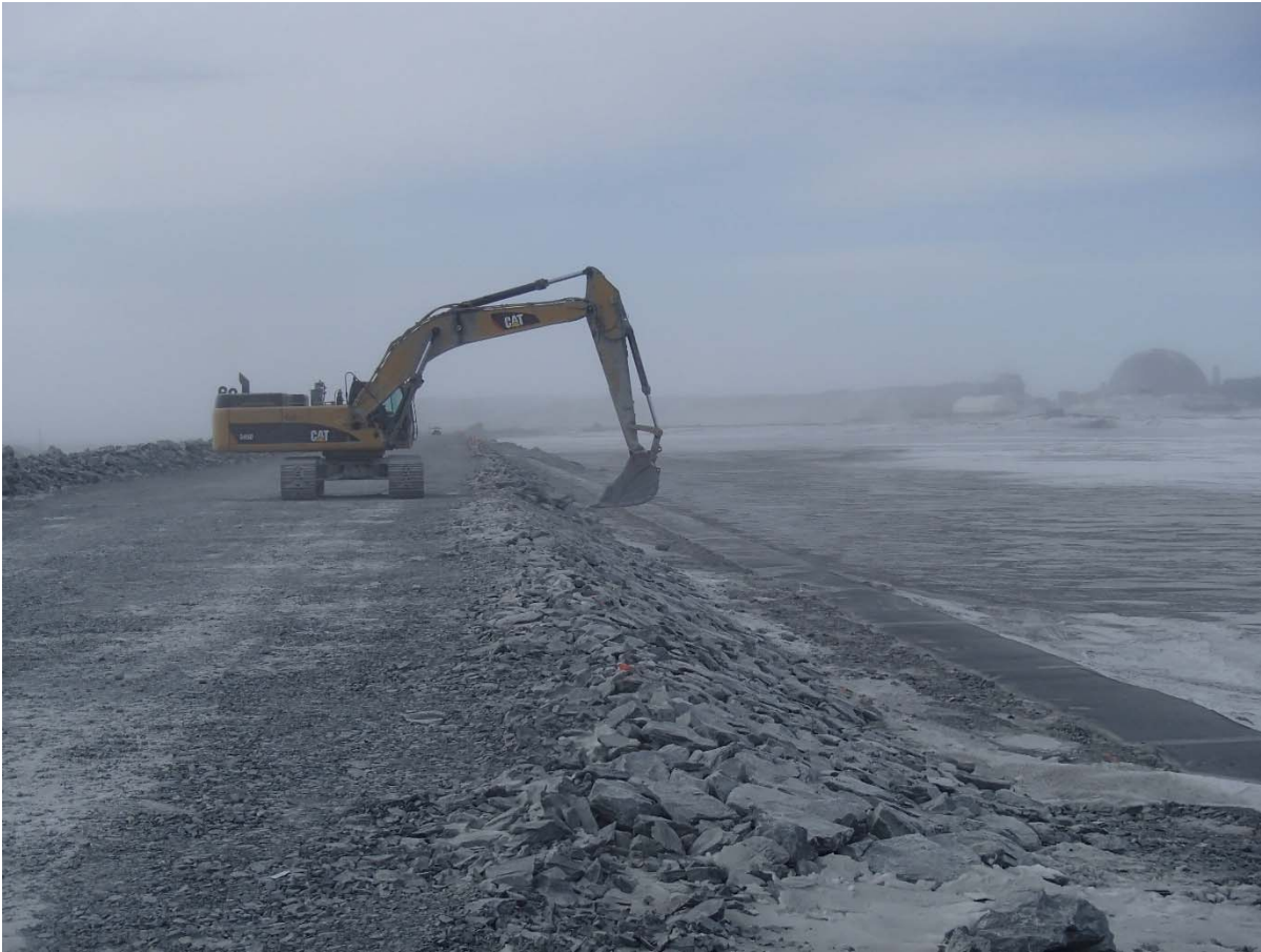
Photograph CD-1816: From Sta. 0+175/-27, looking S. Profiling of the upstream slope (2H:1V) from El. 143 to 145 m with an excavator between Sta. 0+175 and 0+560 m.
