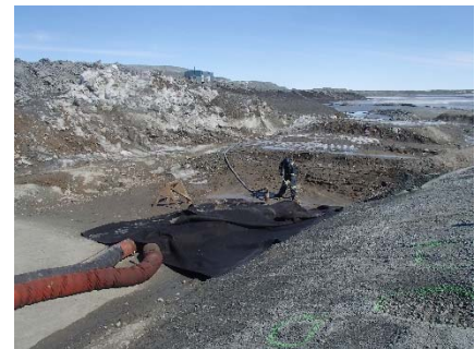
SD3-305 (2018-06-05), looking NE from Sta. 20+590/-48 m. Dewatering of the water ponding on the first compacted sieved till layer of upstream toe liner tie-in. A Genset Frost-fighter is heating the sieved till layer and a pump is evacuating the water.
