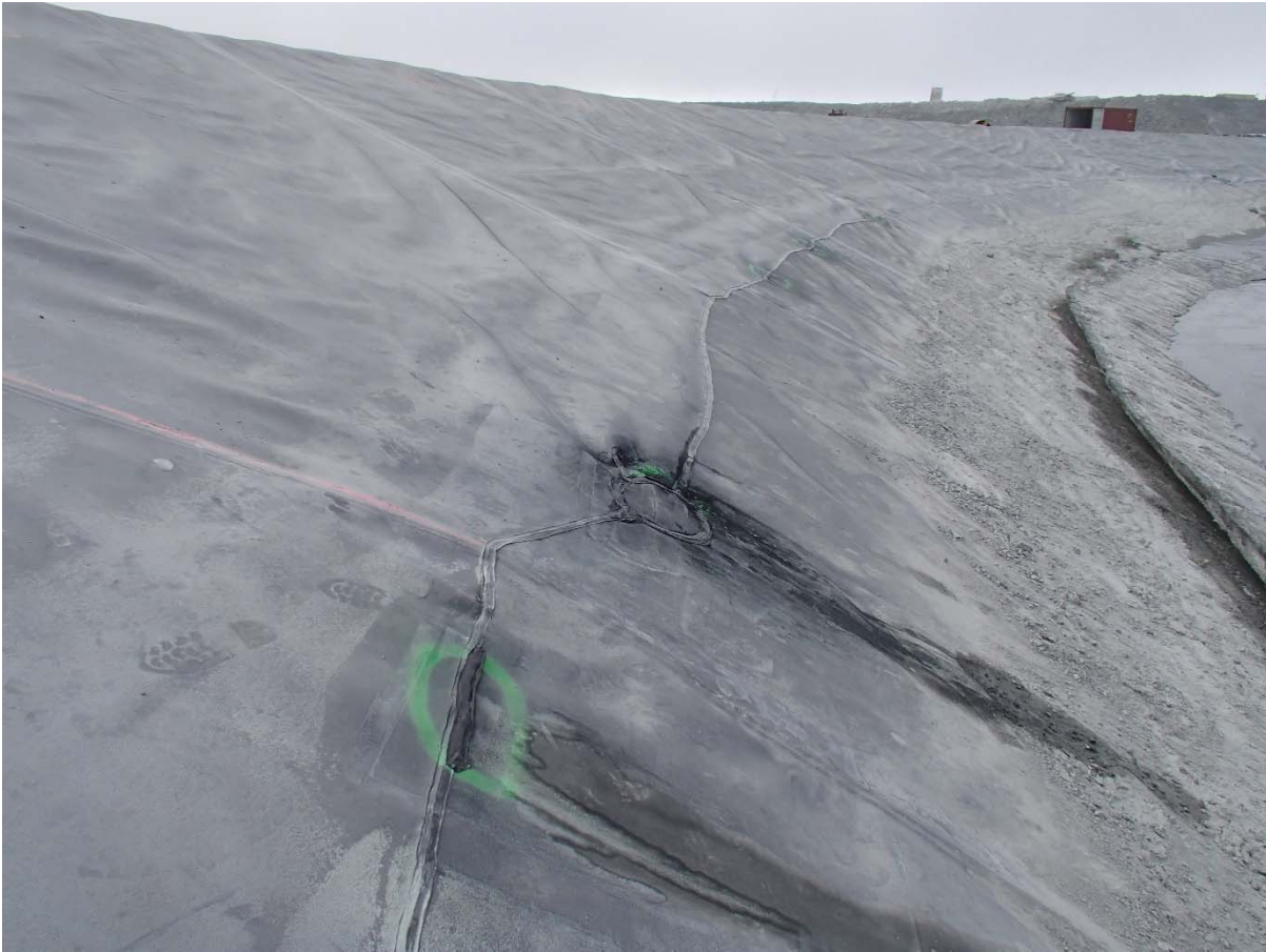
Photograph CD-1893: From Sta. 0+950/-27 m, looking SW. View of repair patches on the extrusion weld at the bottom of panels 803, 807, 808, 810, 814, 815, 816 and 818.
