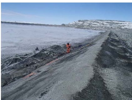
CD-1856 (2018-05-18), looking N from Sta. 0+670/-24 m. Clean-up of the fine filter placed against the slope at the deposition finger at approx. Sta. 0+670 m with pressurized air stream to expose 1 m of LLDPE liner, in preparation for the new liner installation.
