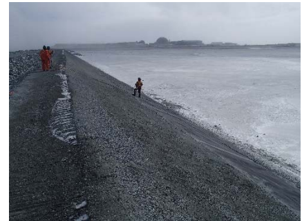
CD-1855 (2018-05-16), looking S from Sta. 0+230/-22 m. Clean-up of the existing LLDPE with pressurized air stream in preparation for liner installation between Sta. 0+170 m and 40+780 m 3 .
