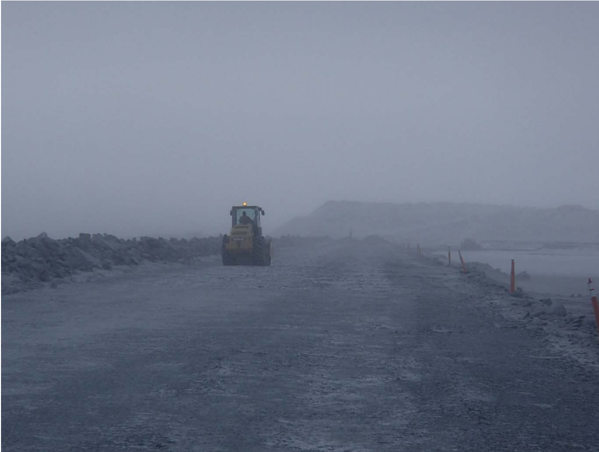
Photograph CD-1810: From Sta. 0+335/-15 m looking S. Compaction of the 2 m lift (approx.) of IV rockfill at El. 145 m with a 10-tonne smooth-drum compactor with vibration (6 passes) from Sta. 0+350 to 0+540 m (o.s. -19 to -7 m).
