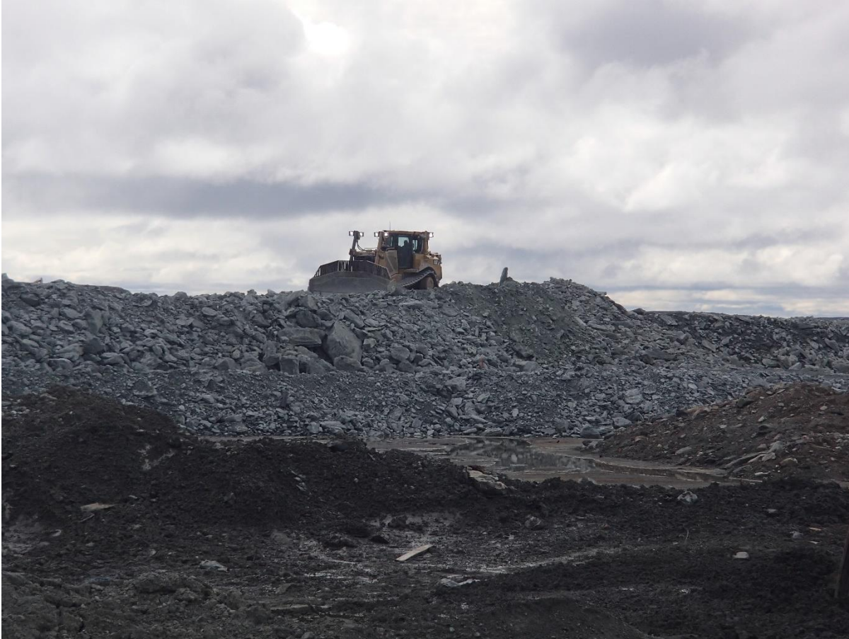
Photograph NCIS-084: From Sta 1+080/+47 m (approx.), looking E. Placement of a 2 m thick (approx.) lift of UM rockfill from El. 150 m to El. 152 m (approx.) with a dozer from Sta. 1+160 m to 1+130 m (-55 m to -102 m).
