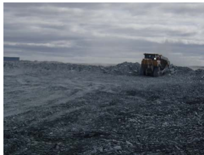
NCIS-044 (2018-06-25), looking S from Sta. 1+200/-19 m. Placement of a 1.5 to 2 m thick (approx.) lift of UM rockfill from El. 148 m to El. 150 m (approx.) with a dozer from Sta. 1+150 m to 1+120 m (-92 m to +10 m). The material is of good quality and is well graded.
