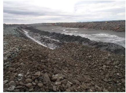
NCIS-138 (2018-08-01), looking SW from Sta. 1+365/+15 m (approx.). Excavation of a 0.8 m (approx.) deep, 1 m wide shallow ditch in the tailings and placement of a 0.3 m thick (approx.) layer of till sieving reject material on the bottom and on the slopes of the ditch from Sta. 1+200 m to 1+100 m.
