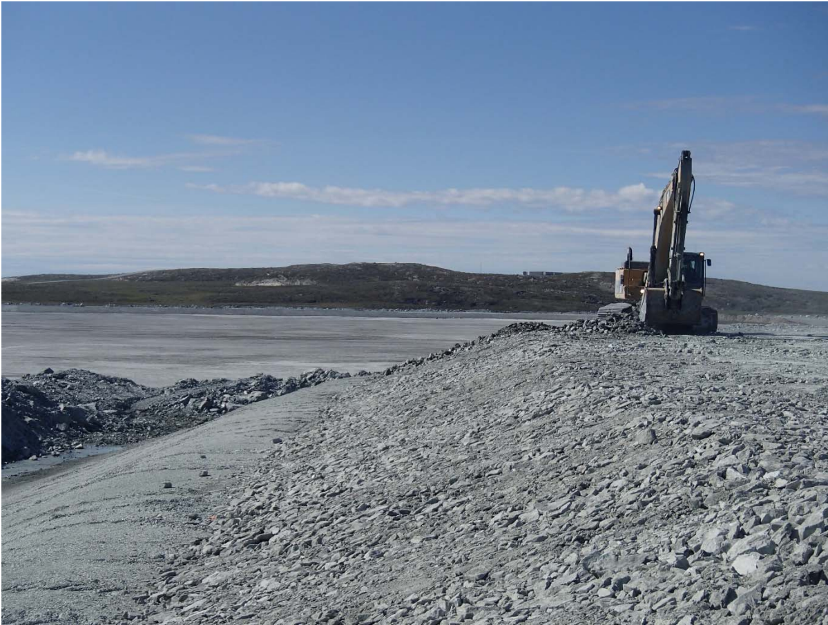
Photograph NCIS-102: From Sta. 2+680/-21 m (approx.), looking W. Placement of a 0.5 m thick lift of coarse filter in the upstream slope from El. 152 m to 154 m with an excavator from Sta. 2+575 m to 2+710 m and from Sta. 2+411 m to 2+460 m.
