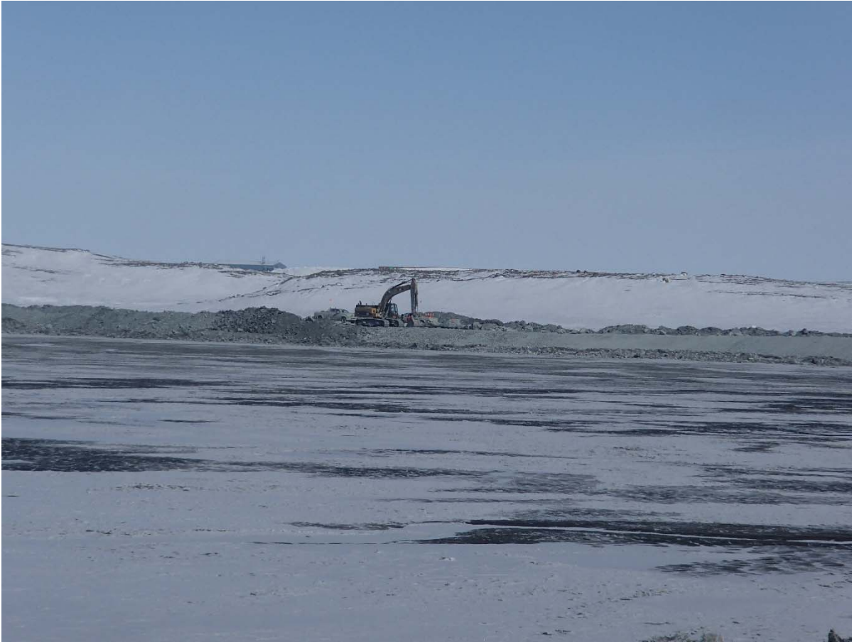
Photograph NCIS-018: From Sta. 2+310 m (approx.), looking NW. Profiling of the upstream slope (3H:1V) from El. 150 to 152 m with an excavator from Sta. 1+989 m to 1+860 m.
