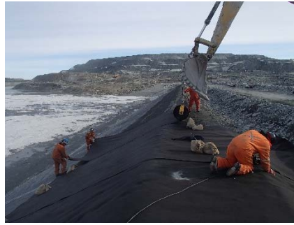
CD-1887 (2018-06-04), looking N from Sta. 0+310/-26 m. Installation of the geotextile on the upstream slope 2H:1V between El. 143 m and 145 m from Sta. 0+320 m to 0+160 m.
