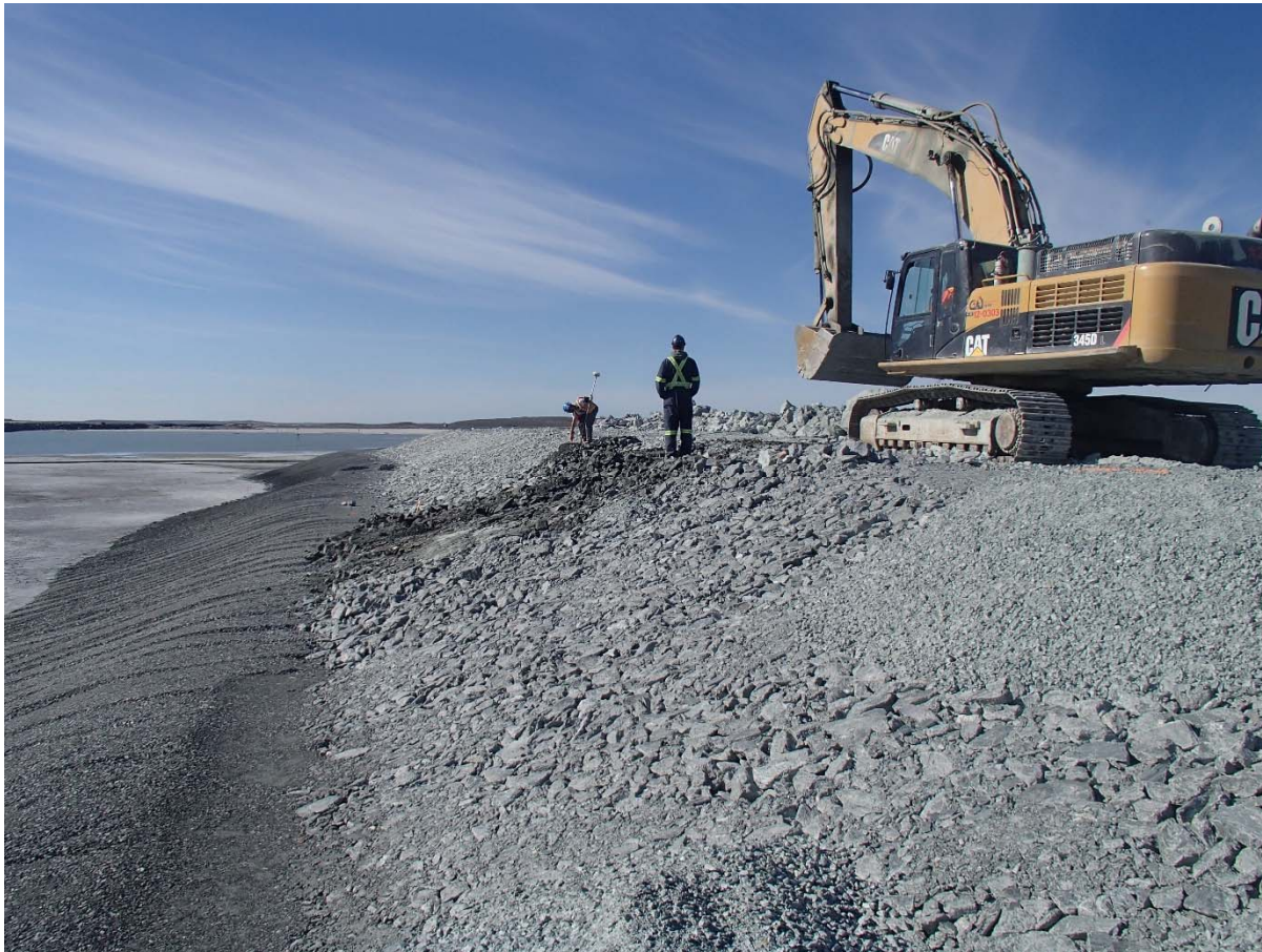
Photograph NCIS-097: From Sta. 1+180/-75 m (approx.), looking SW. Placement of a 0.5 m thick lift of coarse filter in the upstream slope from El. 150 m to 152 m with an excavator from Sta. 1+200 m to 1+113 m.
