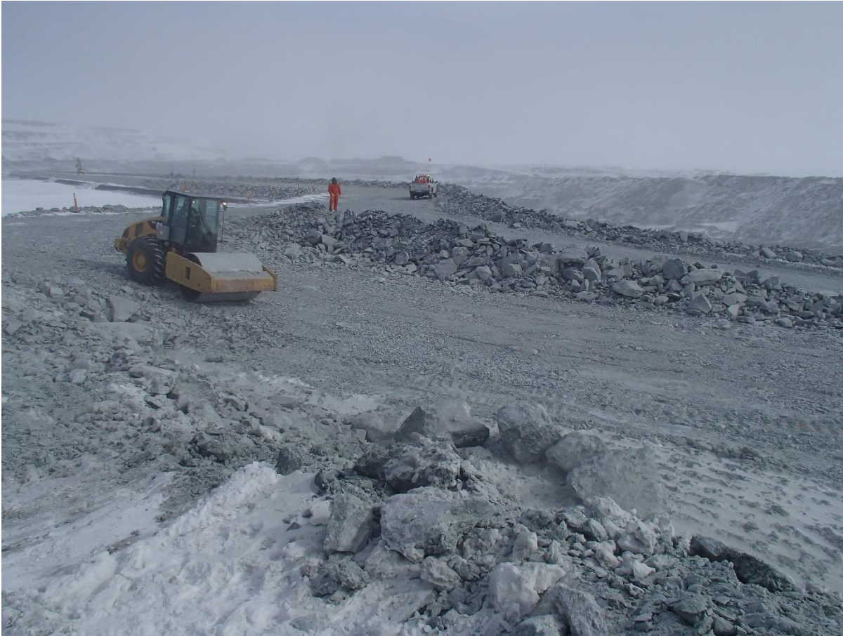
Photograph CD-1823: From Sta. 0+175/+8, looking NE. Compaction of the two 2 m lifts (approx.) of intermediate volcanic (IV) rockfill at El. 143 and at El. 145 m with a 10-tonne smooth-drum compactor with vibration (6 passes) from Sta. 40+720 m to 40+750 m (o.s. -10 to +10 m).
