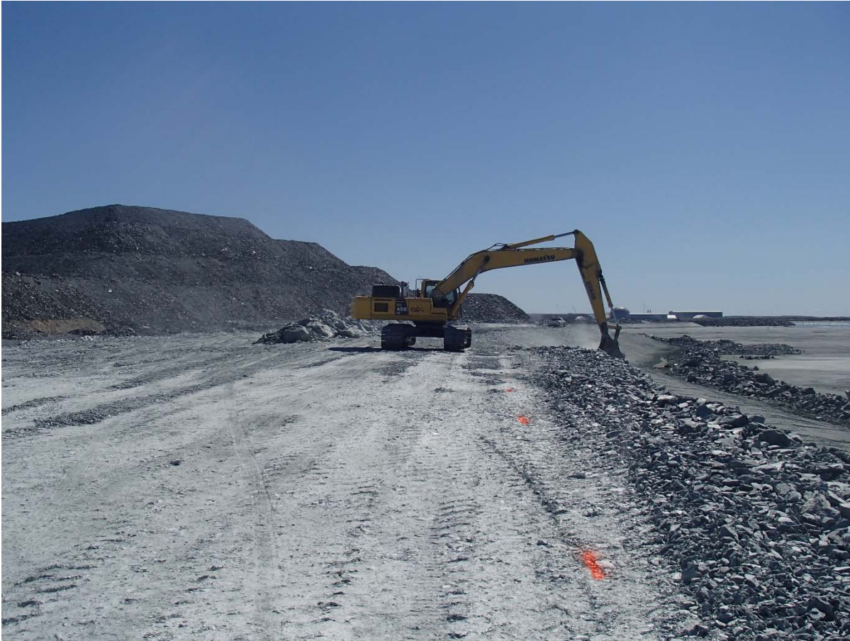
Photograph NCIS-095: From Sta 2+375/-18 m (approx.), looking S. Profiling of the upstream slope (3H:1V) from El. 152 to 154 m with an excavator from Sta. 2+545 m to 2+410 m.
