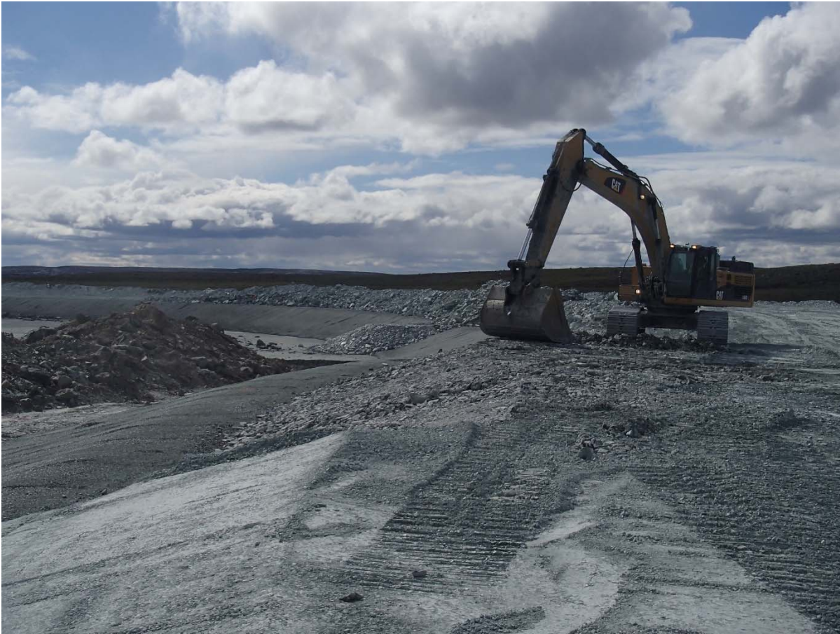
Photograph NCIS-133: From Sta. 1+820/-28 m (approx.), looking W. Placement of a 0.5 m thick lift of coarse filter in the upstream slope from El. 152 m to 154 m with an excavator from Sta. 1+890 m to 1+826 m.
