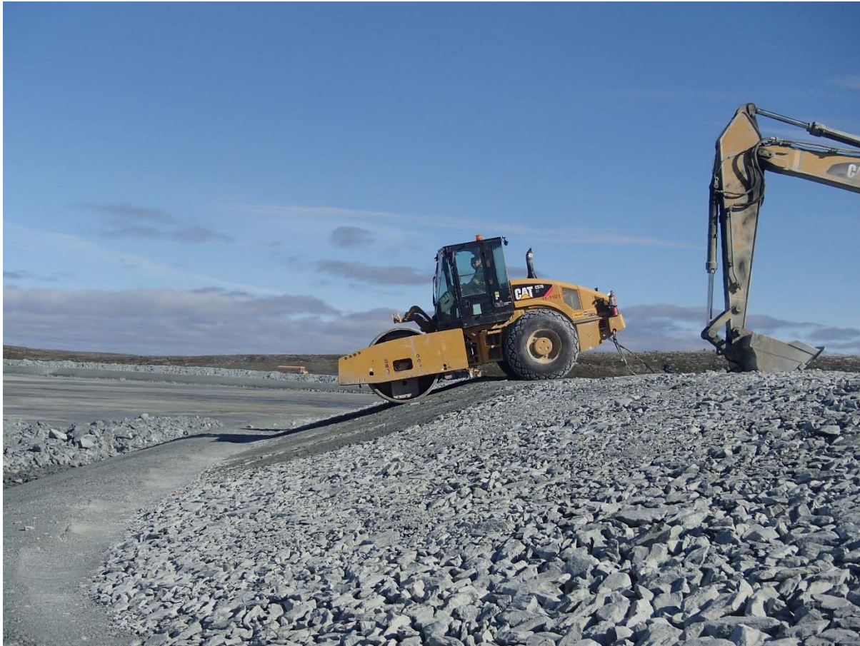
Photograph NCIS-105: From Sta. 2+630/-34 m (approx.), looking NW. Compaction of the 0.5 m lift (approx.) of coarse filter between El. 152 m and 154 m with a 10-tonne smooth-drum compactor with vibration (4 passes) in the upstream slope from Sta. 2+710 m to 2+411 m.
