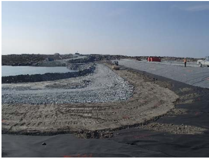
SD3-327 (2018-07-11), looking S from Sta. 20+610/-43 m. Compaction of the 0.5 m lift of low quality till (0-150 mm) at El. 142.5 m with a 10-tonne smooth-drum compactor with vibration (4 passes) from Sta. 20+610 m to 20+615 m and from Sta. 20+635 m to 20+760 m.
