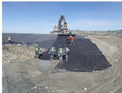
SD3-322 (2018-07-09), looking W from Sta. 20+625/-63 m. Installation of two layers of geotextile on the upstream slope 3H:1V between El. 142 m and 143 m (approx.) from Sta. 20+610 m to 20+800 m.
