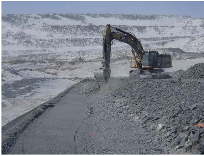
CD-1832 (2018-05-07), looking N from Sta. 0+280/-25 m. Placement of a second 0.5 m thick lift of coarse filter from El. 143.5 m to 144 m with an excavator from Sta. 0+175 m to 0+280 m.
