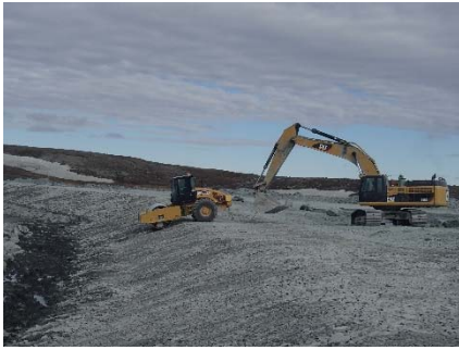
NCIS-037 (2018-06-22), looking NW from Sta. 1+550/-25 m. Compaction of the 0.5 m lift (approx.) of coarse filter between El. 150 and 152 m with a 10-tonne smooth-drum compactor (4 passes) in the upstream slope from Sta. 2+450 to 1+805 m.
