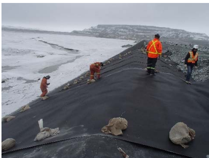
CD-1874 (2018-05-29), looking N from Sta. 0+760/-26 m. Installation of the LLDPE liner on the upstream slope 2H:1V between El. 143 m and 145 m from Sta. 0+760 m to 0+740 m (panel numbers 845 to 848).
