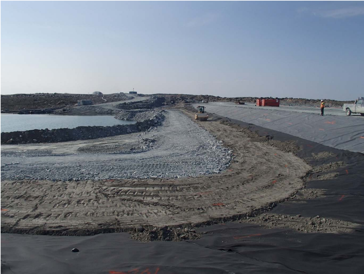
Photograph SD3-327: From Sta. 20+610/-43 m, looking S. Compaction of the 0.5 m lift of low quality till (0-150 mm) at El. 142.5 m with a 10-tonne smooth-drum compactor with vibration (4 passes) from Sta. 20+610 m to 20+615 m and from Sta. 20+635 m to 20+760 m.
