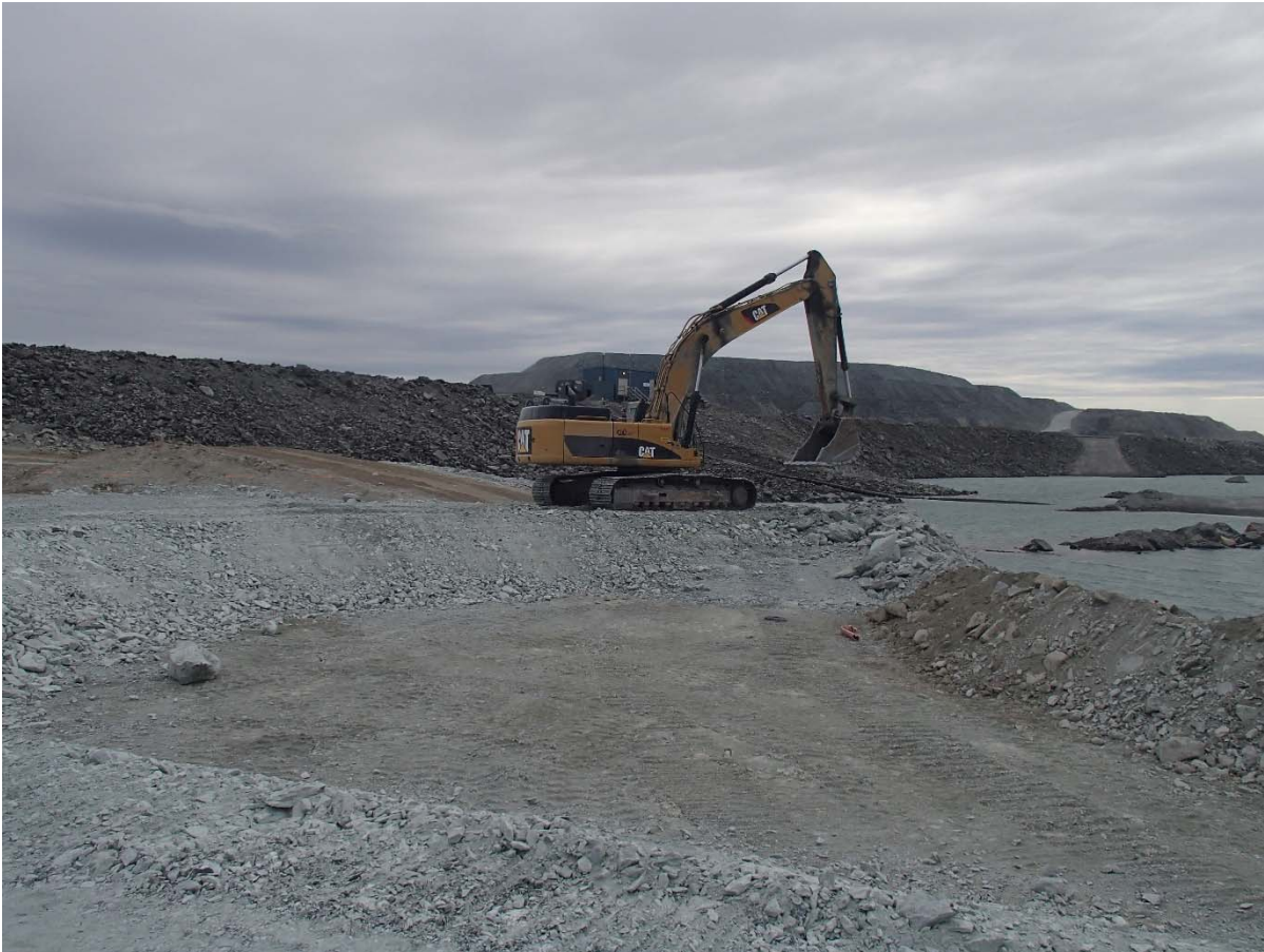
Photograph SD3-347: From Sta. 20+640/-41 m, looking W. Placement of a third 0.5 m thick lift of fine UM rockfill (0-500 mm) upstream of the low quality till (0-150mm) from El. 143 m to 143.5 m from Sta. 20+688 m to 20+619 m.
