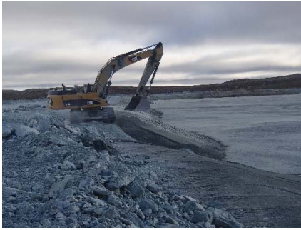
NCIS-073 (2018-07-03), looking N from Sta. 1+300/-33 m. Placement of a 0.5 m thick lift of fine filter over the coarse filter in the upstream slope from El. 150 m to 152 m with an excavator from Sta. 1+320 m to 1+300 m.
