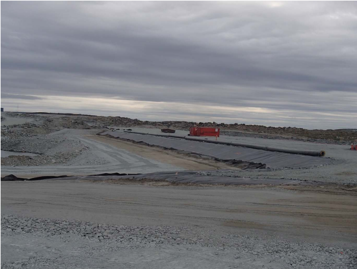
Photograph SD3-353: From Sta. 20+580/-49 m, looking SW. View of SD3 at the end of the 2018 construction phase.
