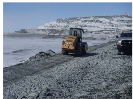
CD-1840 (2018-05-09), looking NW from Sta. 0+575/-15 m. Compaction of the second 0.5 m lift (approx.) of fine and coarse filters material at El. 144 m with a 10-tonne smooth-drum compactor with vibration (4 passes) from Sta 0+500 m to 40+730 m.
