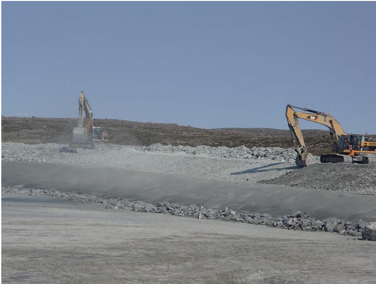
Photograph NCIS-111: From Sta. 2+320/-22 m (approx.), looking NW. Profiling of the upstream slope (3H:1V) from El. 152 to 154 m with an excavator from Sta. 2+159 m to 2+000 m and placement of a 0.5 m thick lift of coarse filter in the upstream slope from El. 152 m to 154 m with an excavator from Sta. 2+293 m to 2+080 m.
