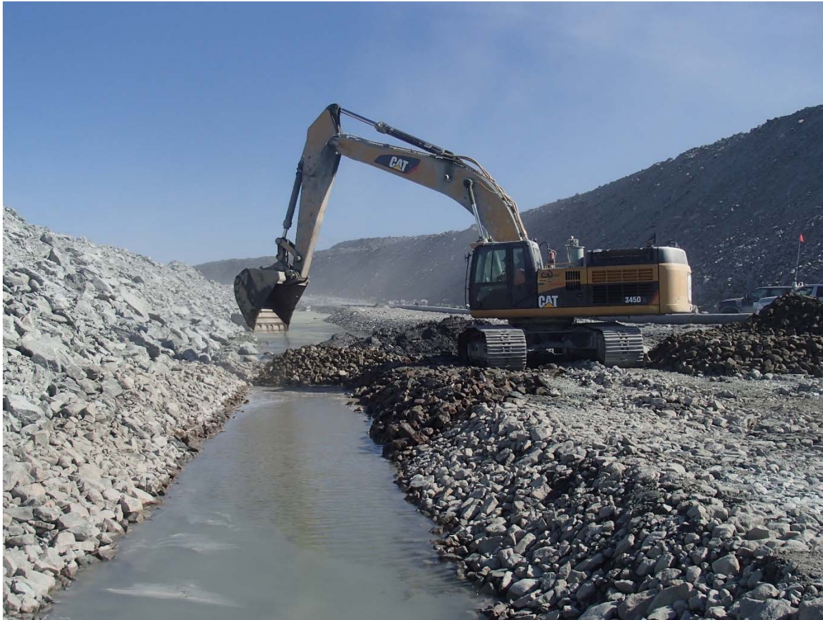
Photograph NCIS-125: From Sta. 3+050/+26 m (approx.), looking NE. Corrections to the north sump: removal of approx. 0.5 m of tailing and till sieving reject material on the bottom of the excavation. The erosion protection material was replaced.
