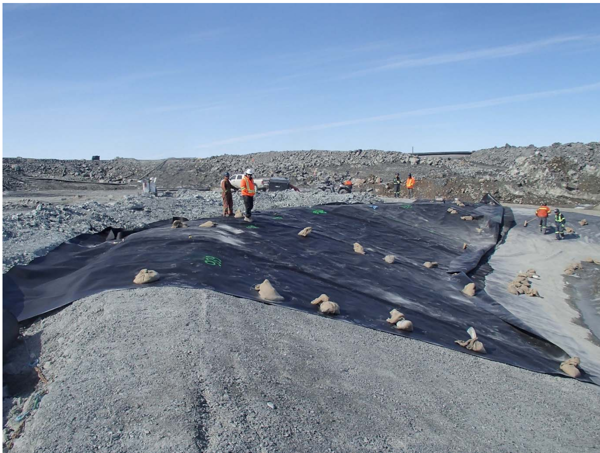
Photograph SD3-309: From Sta. 20+640/-26 m, looking N. Installation of the LLDPE liner on the upstream slope 3H:1V between El. 143 m and 145 m from Sta. 20+610 m to 20+810 m (panel numbers 934 to 964).
