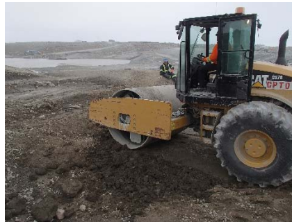
SD3-313 (2018-06-08), looking S from Sta. 20+600/-52 m. Compaction of the 0.15 m-thick lift of compacted sieved till with a 10-tonne smooth-drum compactor without vibration (4 passes) from Sta. 20+596 m to 20+601 m.
