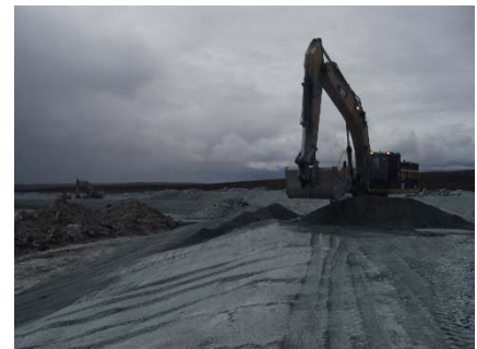
NCIS-135 (2018-07-30), looking SW from Sta. 1+860/-12 m (approx.). Placement of a 0.5 m thick lift of fine filter in the upstream slope from El. 152 m to 154 m with an excavator from Sta. 1+830 m to 1+700 m.
