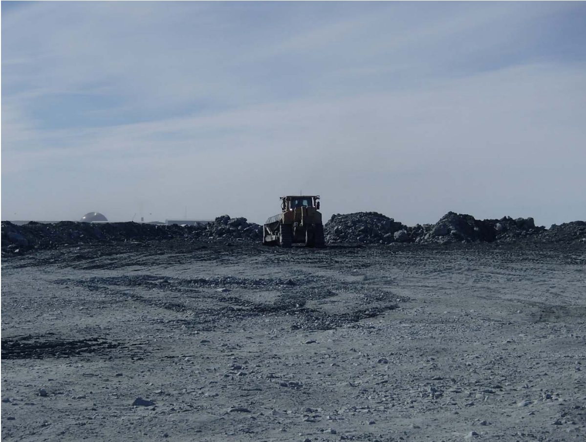
Photograph NCIS-026: From Sta. 1+440/+2 m, looking S. Placement of a 2 m thick (approx.) lift of UM rockfill from El. 150 m to El. 152 m (approx.) with a dozer from Sta. 1+390 m to 1+365 m (offset +10 m to -29 m).
