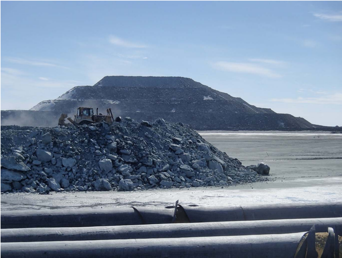
Photograph NCIS-027: From Sta. 1+360/+67 m, looking S. Placement of a 2 m thick (approx.) lift of UM rockfill from El. 150 m to El. 152 m (approx.) with a dozer from Sta. 1+365 m to 1+360 m (offset +9 m to -28 m).
