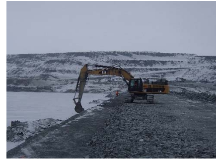
CD-1846 (2018-05-12), looking N from Sta. 0+835/-25 m. Profiling of the upstream slope (2H:1V) from El. 143 to 145 m with an excavator between Sta. 0+330 and 0+600 m and between Sta. 0+715 m and 40+730 m.
