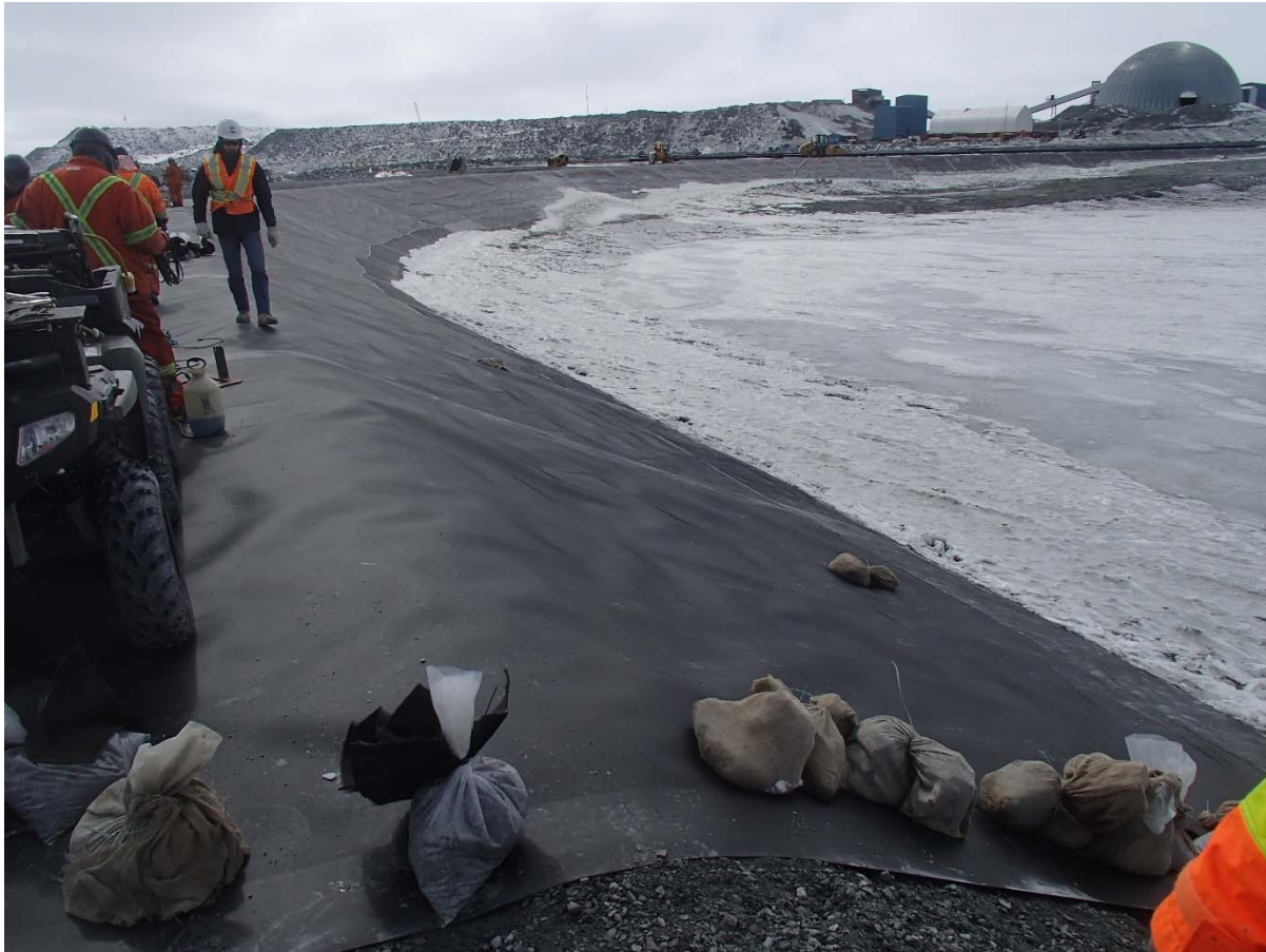
Photograph CD-1870: From Sta. 0+900/-26 m, looking S. Installation of the LLDPE liner on the upstream slope 2H:1V between El. 143 m and 145 m from Sta. 0+935 m to 0+900 m (panel numbers 820 to 823).
