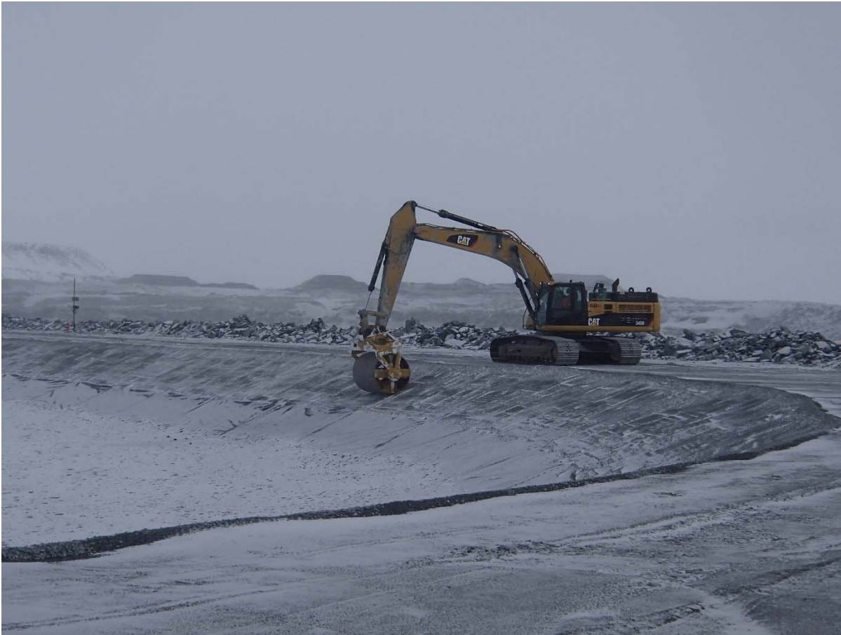
Photograph CD-1849: From Sta. 40+750/-17 m, looking NE. Final rolling of the upstream slope in view of the LLDPE geomembrane installation from Sta. 0+170 m to 40+730 m.
