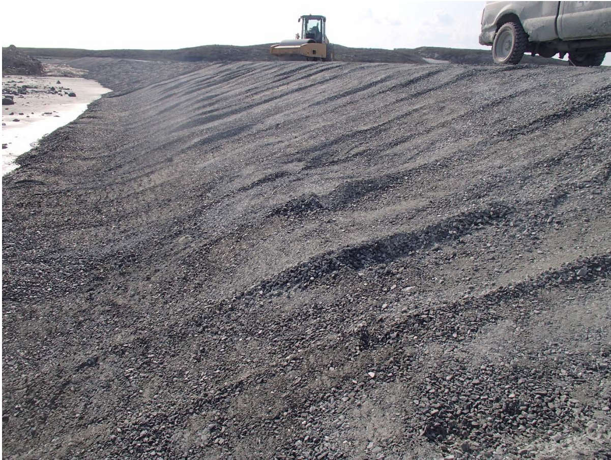
Photograph NCIS-087: From Sta 1+950/-34 m (approx.), looking W. Compaction of the 0.5 m lift (approx.) of fine filter between El. 150 and 152 m with a 10-tonne smooth-drum compactor (4 passes) in the upstream slope from Sta. 2+000 m to 1+930 m. Vibration is used except for the first pass down the slope in order to stabilize the material and limit deformation of the lift.
