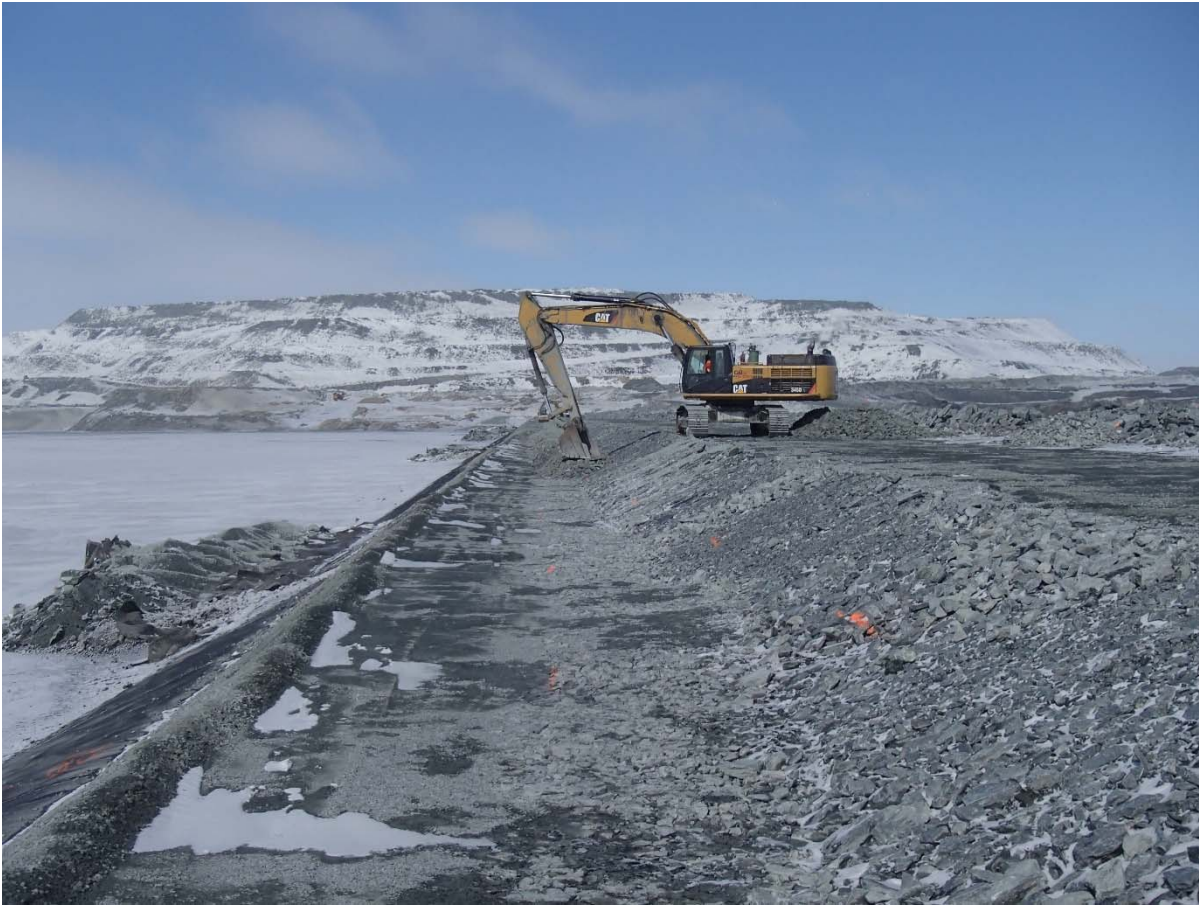
Photograph CD-1838: From Sta. 0+835/-20 m, looking N. Placement of a second 0.5 m thick lift of coarse filter from El. 143.5 m to 144 m with an excavator from Sta. 0+500 m to 0+835 m and from Sta. 0+930 to 40+730 m.
