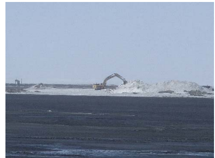
NCIS-024 (2018-05-31), looking SW from Sta. 2+570 m. Removal of the snow bank in the footprint with an excavator from Sta. 1+160 m to 1+120 m (approx.).
