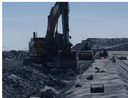
CD-1884 (2018-06-02), looking S from Sta. 0+530/-25 m. Backfilling of the geosynthetic tie-in from Sta. 0+610 m to 0+480 m and compaction of the tie-in material with a 10-tonne smooth-drum compactor with vibration (4 passes) from Sta. 0+610 to 0+480 m.
