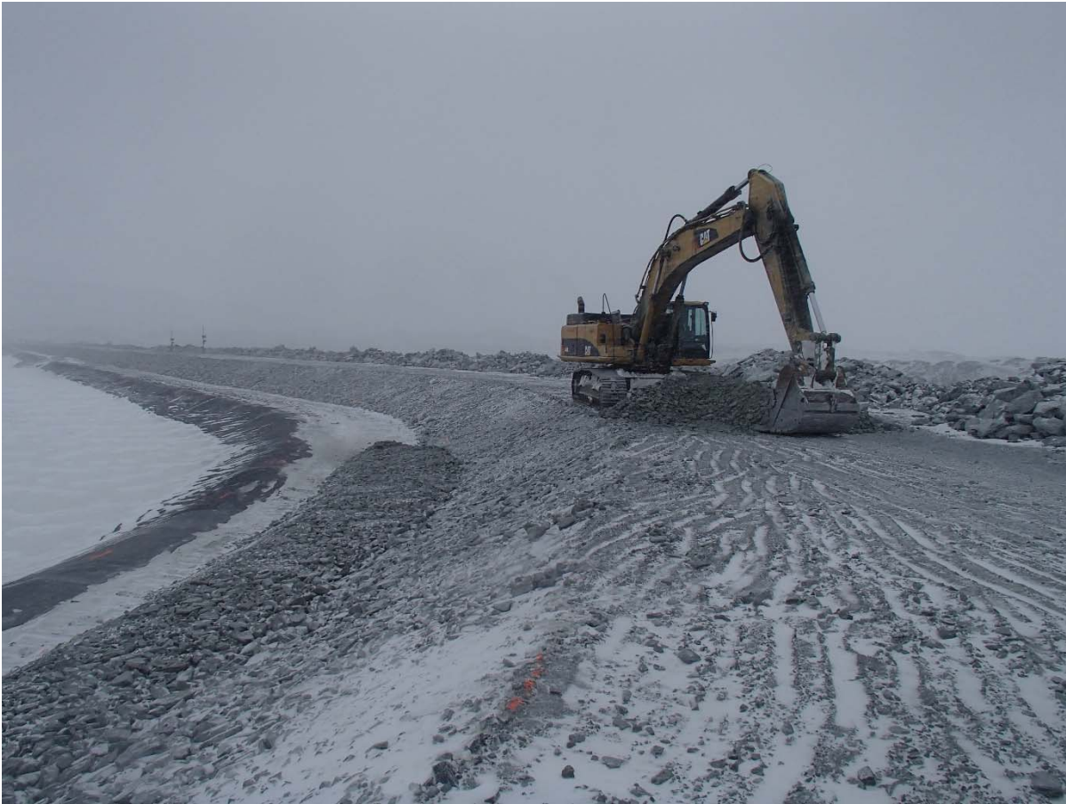
Photograph CD-1826: From Sta 40+770/-27 m, looking NE. Placement of a 0.5 m thick lift of coarse filter from El. 143 m to 143.5 m with an excavator from Sta. 40+730 m to 0+ 775 m.
