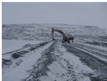
CD-1857 (2018-05-21), looking N from Sta. 0+700/-20 m. Snow removal in the anchoring trench with an excavator between Sta. 0+170 m and 40+780 m.
