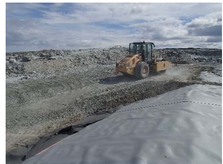
SD3-349 (2018-07-18), looking SE from Sta. 20+765/-29 m. Compaction of the 0.5 m thick lift of fine filter on the top of the upstream toe liner tie-in with a 10 tonne smooth-drum compactor with vibration (4 passes) from Sta. 20+777 m to 20+807 m.
