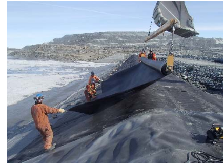
CD-1888 (2018-06-04), looking N from Sta. 0+325/-26 m. Installation of the LLDPE liner on the upstream slope 2H:1V between El. 143 m and 145 m from Sta. 0+320 m to 0+160 m (panel numbers 911 to 910).
