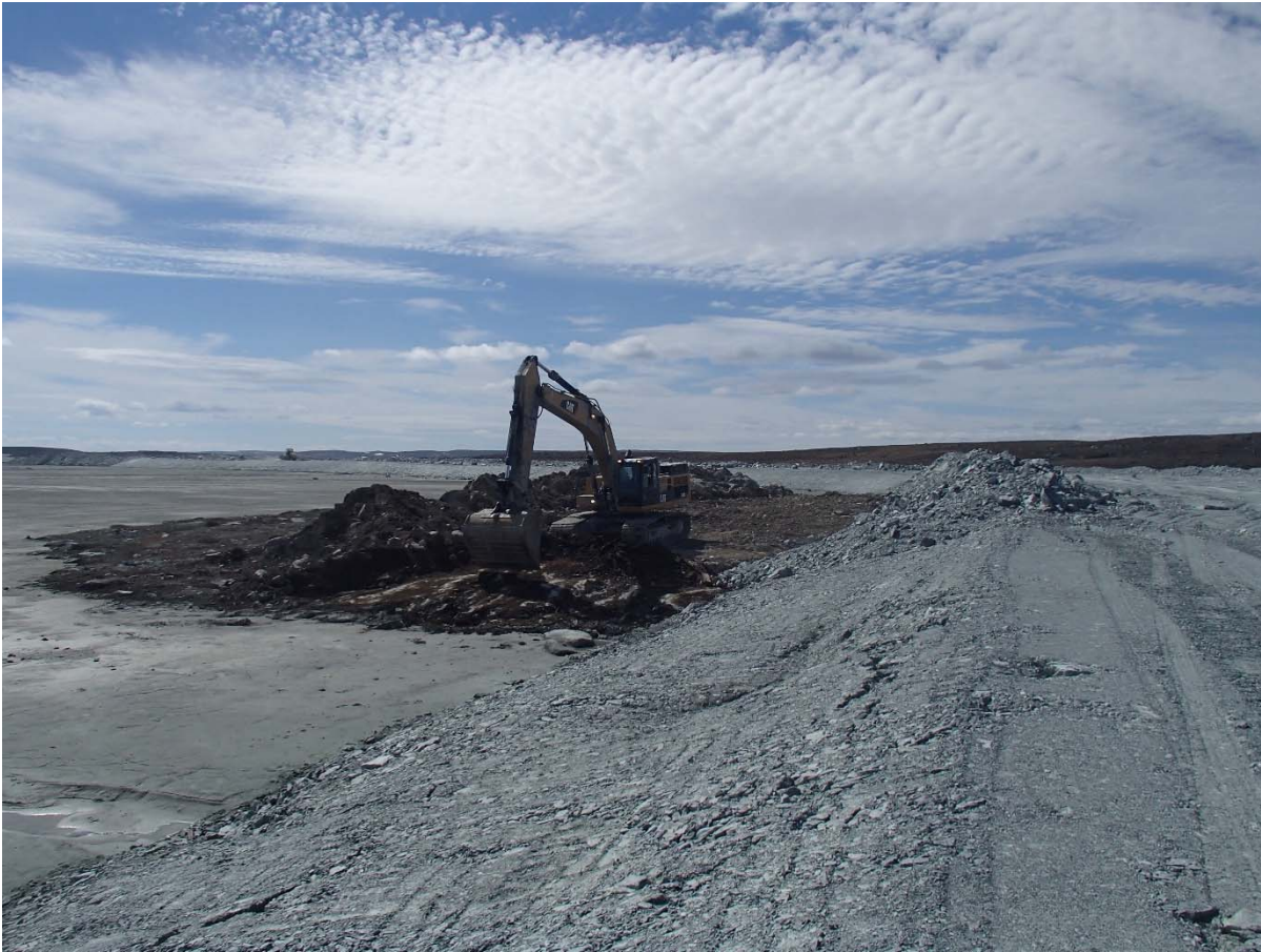
Photograph NCIS-031: From Sta. 1+880/-21 m (approx.), looking SW. Final clean-up of the dike footprint with an excavator to reach a good quality bedrock from Sta. 1+800 to 1+850 m (o.s. -42 to -33 m).
