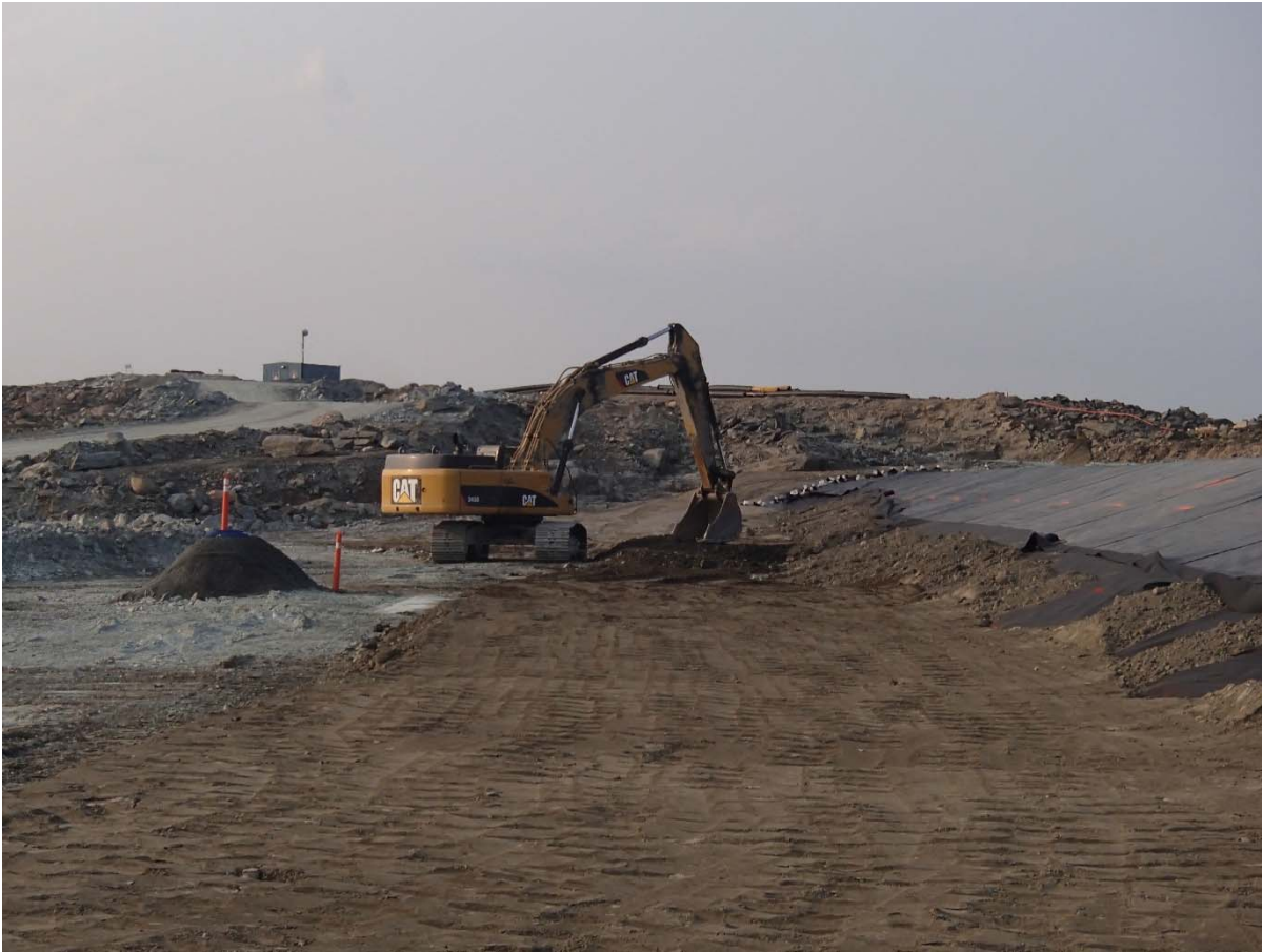
Photograph SD3-324: From Sta. 20+680/-39m, looking S. Placement of a 0.5 m thick lift of low quality till (0-150 mm) from El. 142 m to 142.5 m from Sta. 20+715 m to 20+760 m.
