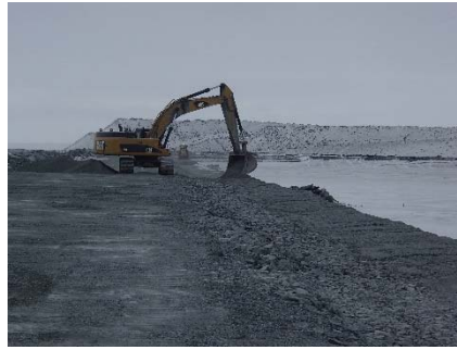
CD-1842 (2018-05-10), looking S from Sta. 0+380/-16 m. Placement of a third 0.5 m thick lift of fine filter from El. 143.5 m to 144 m upstream of the coarse filter with an excavator from Sta. 0+335 m to 0+940 m.
