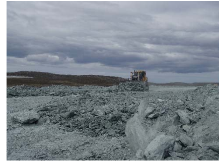
NCIS-069 (2018-07-01), looking NW from Sta. 1+180/-56 m. Placement of a 2 m thick (approx.) lift of UM rockfill from El. 150 m to El. 152 m (approx.) with a dozer from Sta. 1+235 m to 1+160 m (-60 m to -44 m). The material is of good quality and is well graded.
