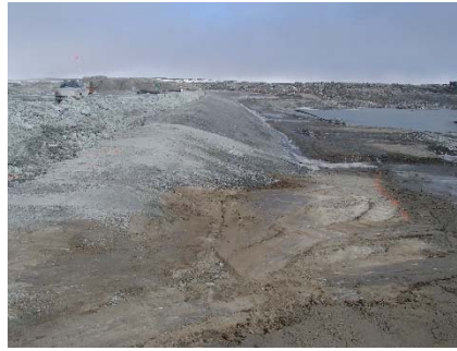
SD3-307 (2018-06-06), looking N from Sta. 20+800/-25 m. View of the liner bedding ready for geosynthetics
