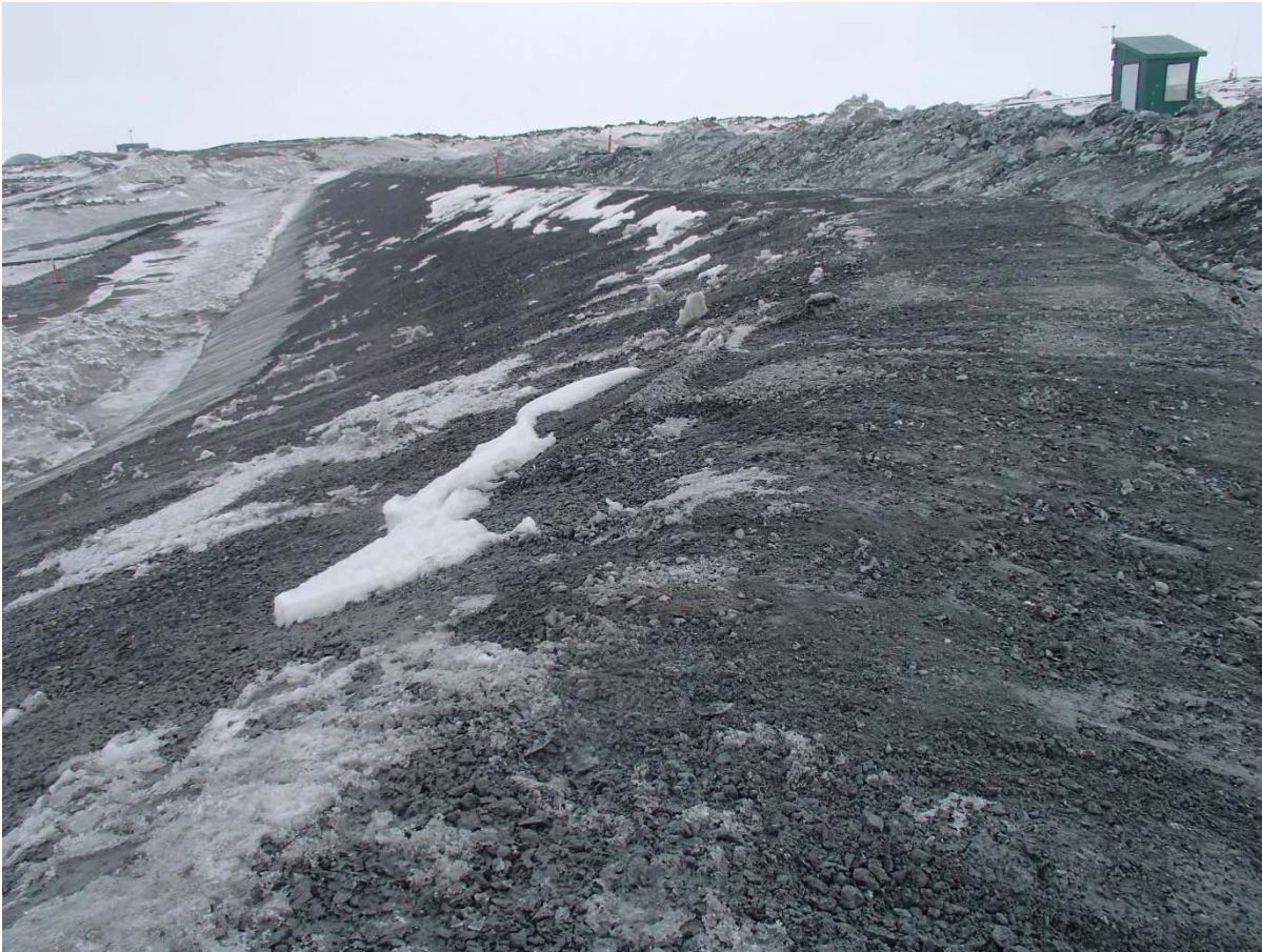
Photograph SD3-304: From Sta. 20+620/-36 m, looking SE. Smoothing of the surface of the fine filter with an excavator on top of the upstream slope from Sta. 20+600 m to 20+780 m.
