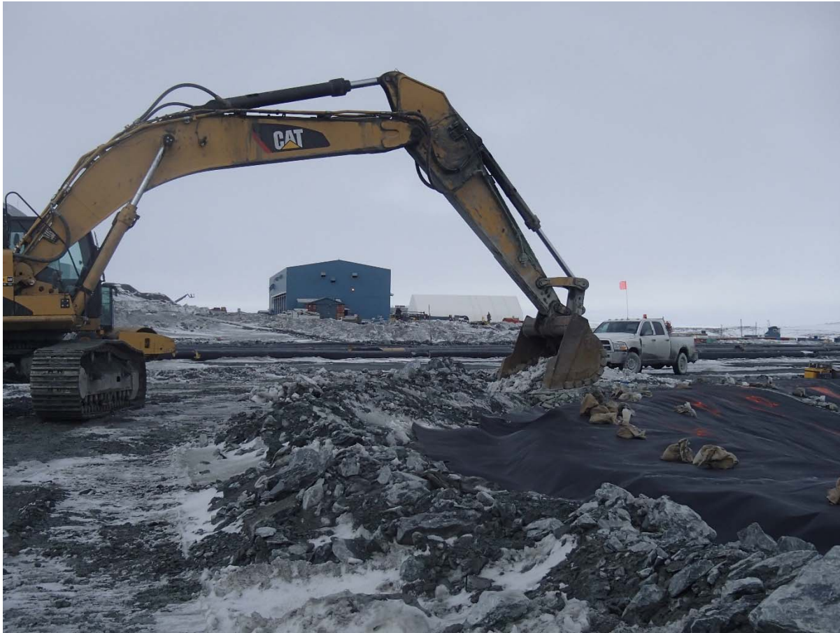
Photograph CD-1863: From Sta. 40+750/-18 m, looking SW. Backfilling of the geosynthetics tie-in from Sta. 40+680 m to 0+950 m.
