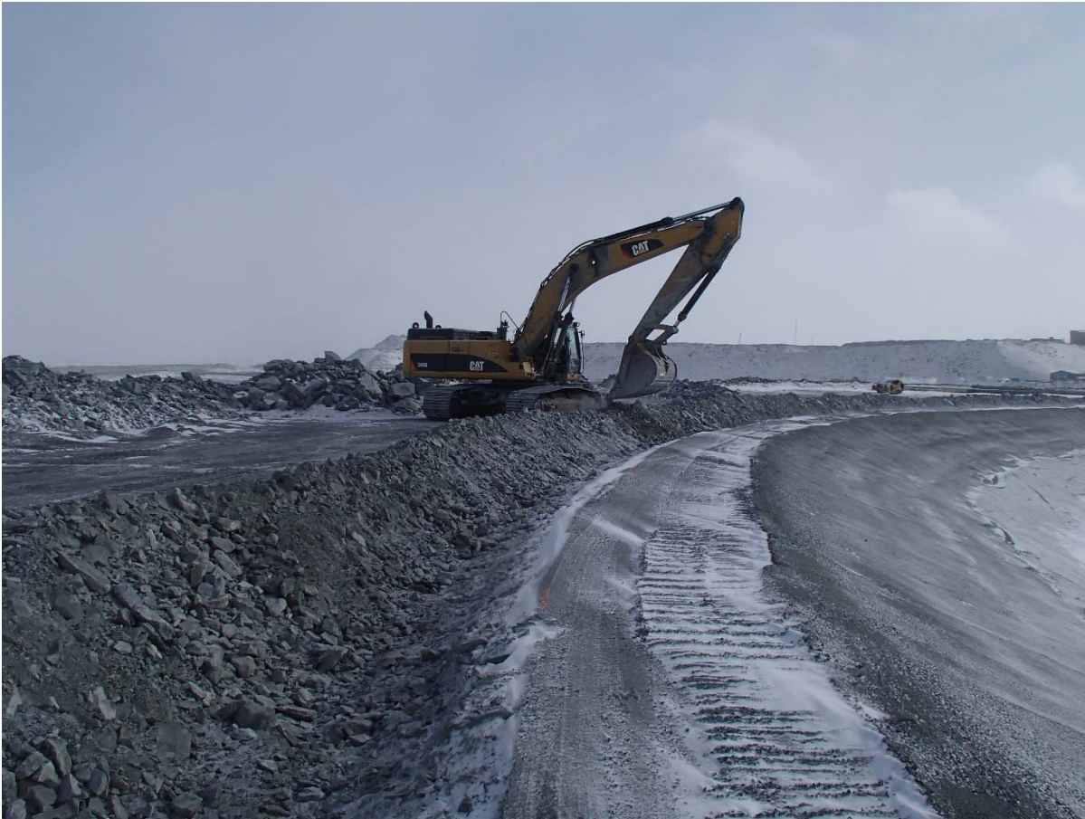
Photograph CD-1851: From Sta. 0+910/-18 m, looking S. Excavation of the LLDPE geomembrane crest anchoring trench from Sta. 40+730 m to 0+830 m.
