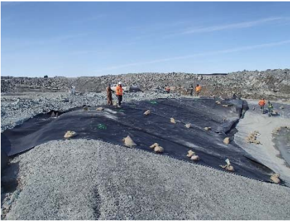
SD3-309 (2018-06-06), looking N from Sta. 20+640/-26 m. Installation of the LLDPE liner on the upstream slope 3H:1V between El. 143 m and 145 m from Sta. 20+620 m to 20+630 m (panel numbers 934 to 939).
