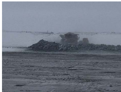
NCIS-008 (2018-05-20). Placement a 2 m thick (approx.) lift of UM rockfill from El. 150 m to El. 152 m (approx.) with a dozer. The material is of good quality and is well graded.
