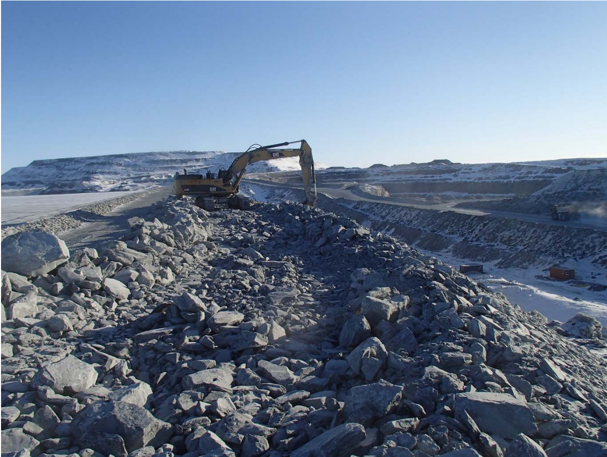
Photograph CD-1854: From Sta. 0+960/-13 m, looking N. Profiling of the downstream slope (1.5H:1V) from El. 143 to 145 m with an excavator between Sta. 0+940 m and 0+990 m.
