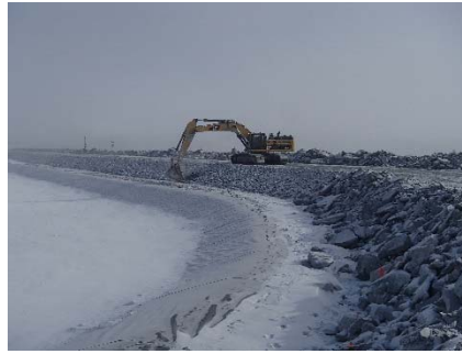
CD-1824 (2018-05-05), looking NE from Sta. 40+760/-25 m. Profiling of the upstream slope (2H:1V) from El. 143 to 145 m with an excavator between Sta. 0+830 m and 40+730 m.
