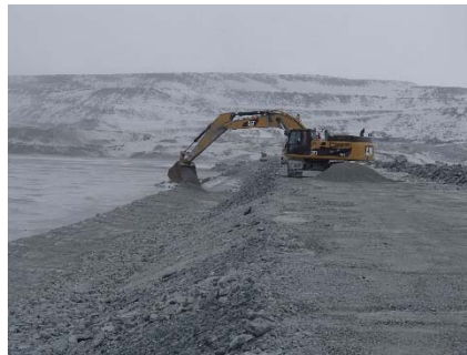
CD-1836 (2018-05-08), looking N from Sta. 0+580/-18 m. Placement of a first 0.5 m thick lift of fine filter from El. 143 m to 143.5 m upstream of the coarse filter with an excavator from Sta. 0+490 m to 0+835 m.
