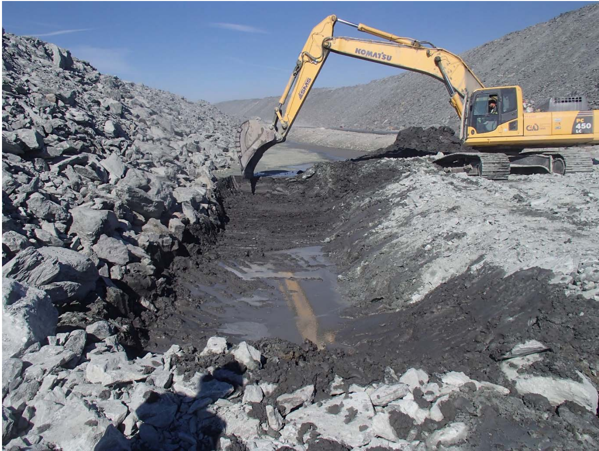
Photograph NCIS-115: From Sta. 3+040/33 m (approx.), looking NE. Excavation of a 1 m (approx.) sump in the tailings with an excavator from Sta. 3+010 m to 3+030 m (o.s. +27 to +30 m). The bottom of the excavation was frozen.
