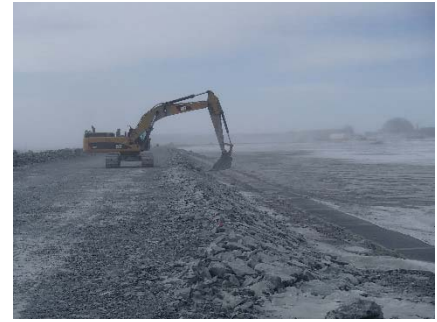
CD-1816 (2018-05-02), looking S from Sta. 0+175/-27 m. Profiling of the upstream slope (2H:1V) from El. 143 to 145 m with an excavator between Sta. 0+175 and 0+560 m.
