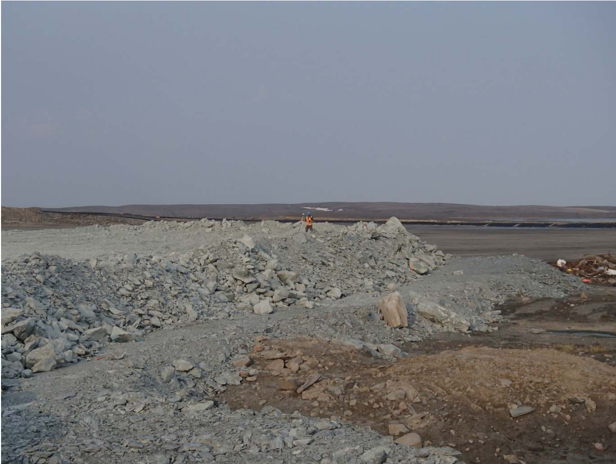
Photograph NCIS-085: From Sta 1+150/-67m (approx.), looking SW. Placement of a 2 m thick (approx.) lift of UM rockfill from El. 150 m to El. 152 m (approx.) with a dozer from Sta. 1+130 m to 1+100 m (-55 m to -78 m).
