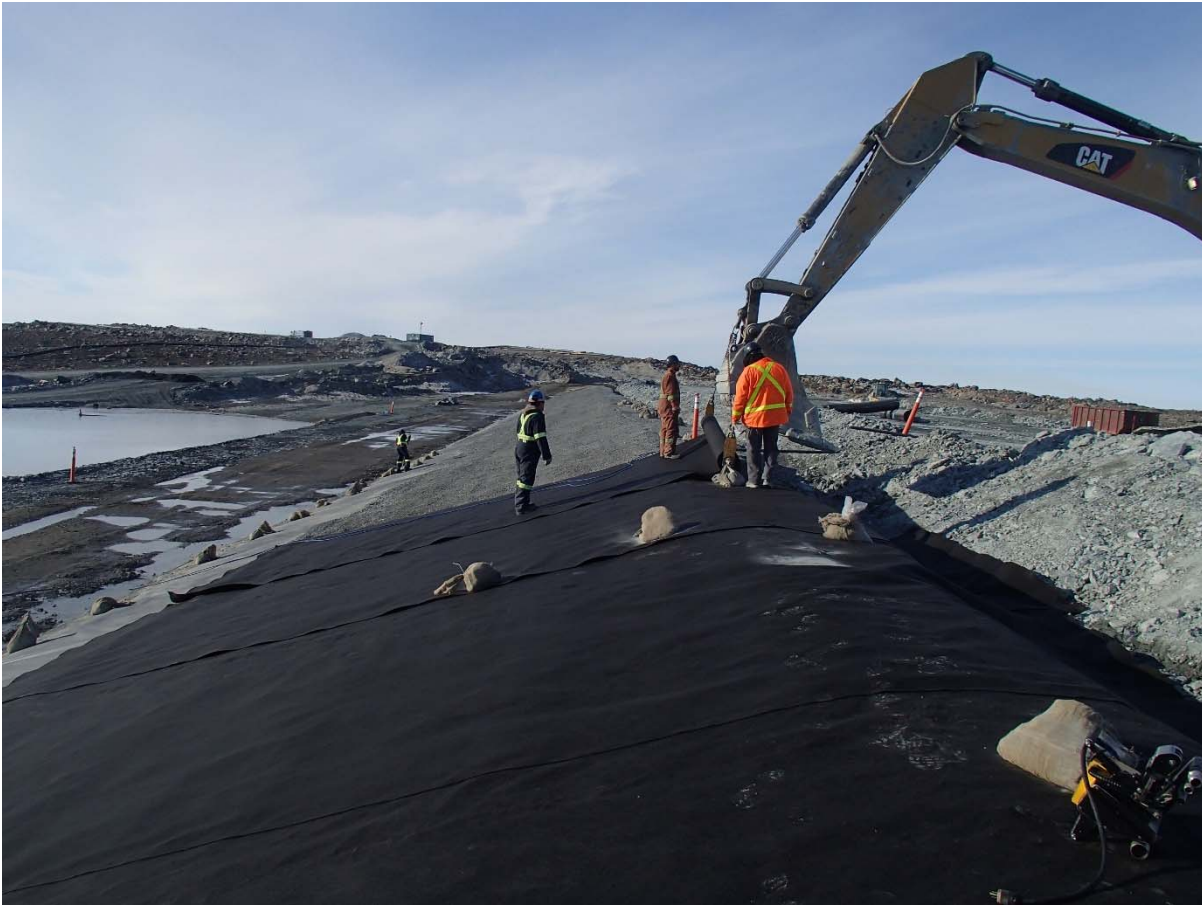
Photograph SD3-310: From Sta. 20+635/-24 m, looking S. Installation of the geotextile on the upstream slope 3H:1V between El. 143 m and 145 m from Sta. 20+630 m to 20+800 m.
