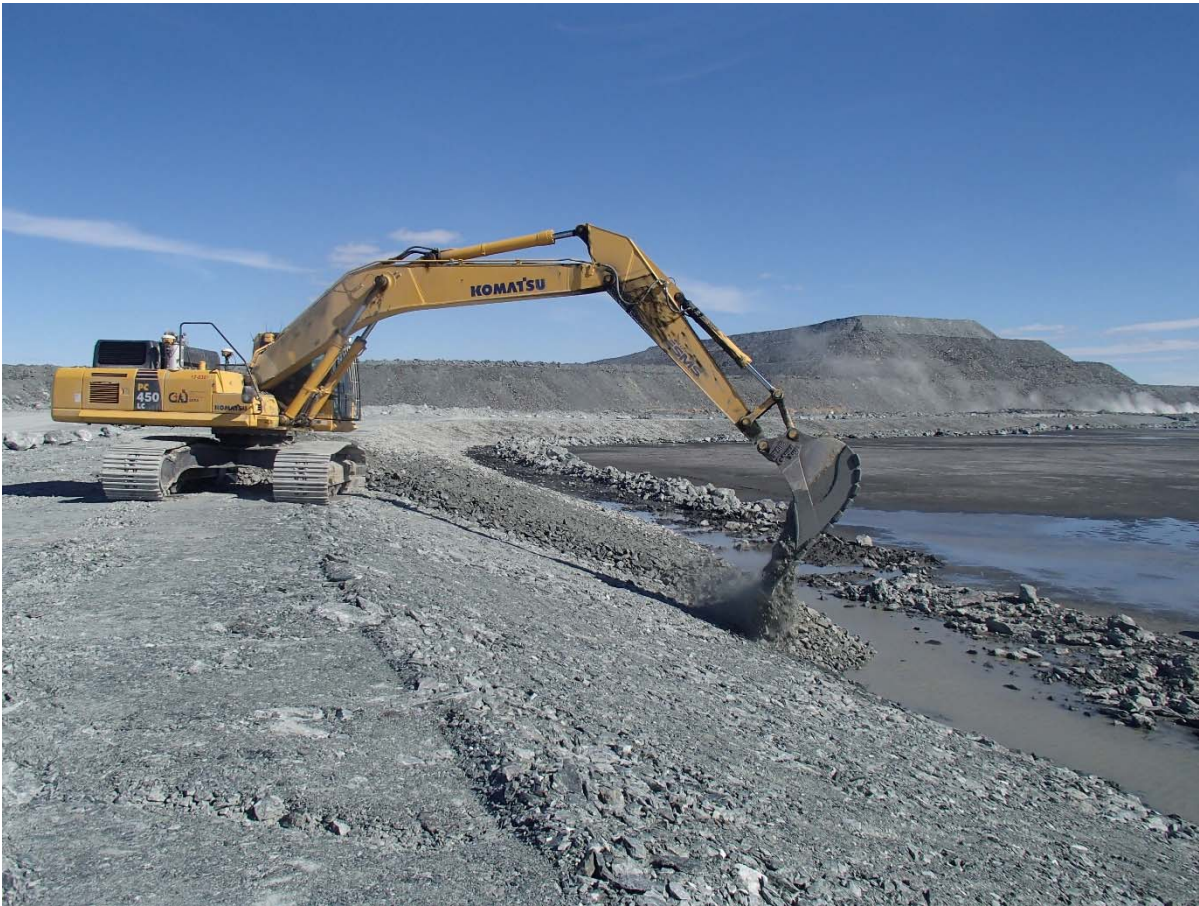
Photograph NCIS-029: From Sta. 2+120/-27 m (approx.), looking SE. Placement of a 0.5 m thick lift of coarse filter in the upstream slope from El. 150 m to 152 m with an excavator from Sta. 2+280 m to 2+105 m.
