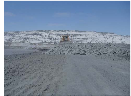
CD-1801 (2018-04-26), looking N from Sta. 0+650/-10 m. Placement a 2 m thick (approx.) lift of intermediate volcanic (IV) rockfill from El. 143 m to El. 145 m from 0+535 to 0+625m (o.s. -28 to -18 m).
