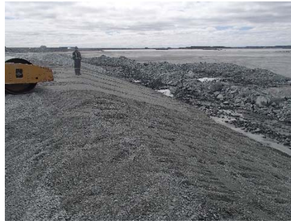
NCIS-038 (2018-06-22), looking SE from Sta. 2+510/-28 m. Compaction of the 0.5 m lift (approx.) of fine filter between El. 150 and 152 m with a 10-tonne smooth-drum compactor (4 passes) in the upstream slope from Sta. 2+542 m to 2+475 m.
