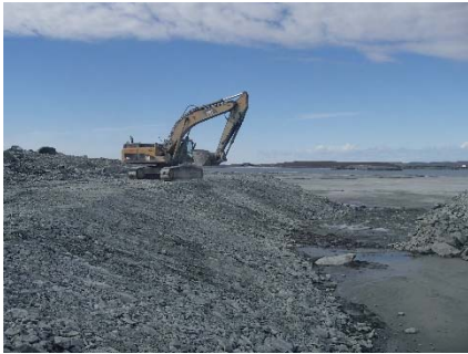
NCIS-067 (2018-07-01), looking N from Sta. 2+880/-26 m. Profiling of the upstream slope (3H:1V) from El. 150 to 152 m with an excavator from Sta. 2+860 m to 2+975 m.
