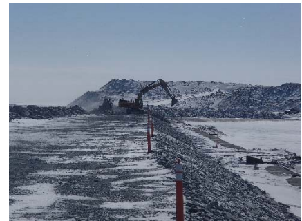
CD-1819 (2018-05-03), looking S from Sta. 0+560/-21 m. Profiling of the upstream slope (2H:1V) from El. 143 to 145 m with an excavator between Sta. 0+560 m and 0+830 m.
