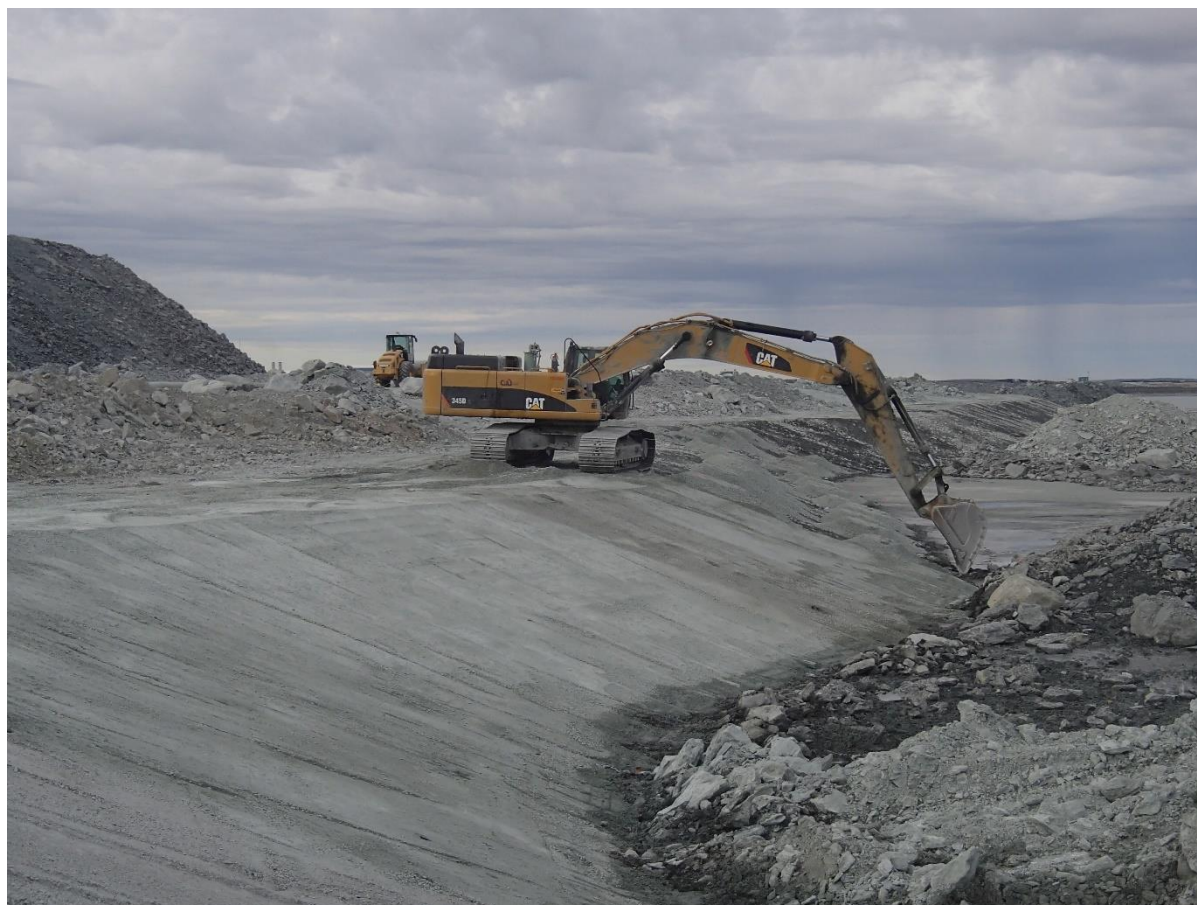
Photograph NCIS-078: From Sta. 2+760/-39 m (approx.), looking S. Placement of a 0.5 m thick lift of fine filter over the coarse filter in the upstream slope from El. 150 m to 152 m with an excavator from Sta. 2+800 m to 2+980 m.
