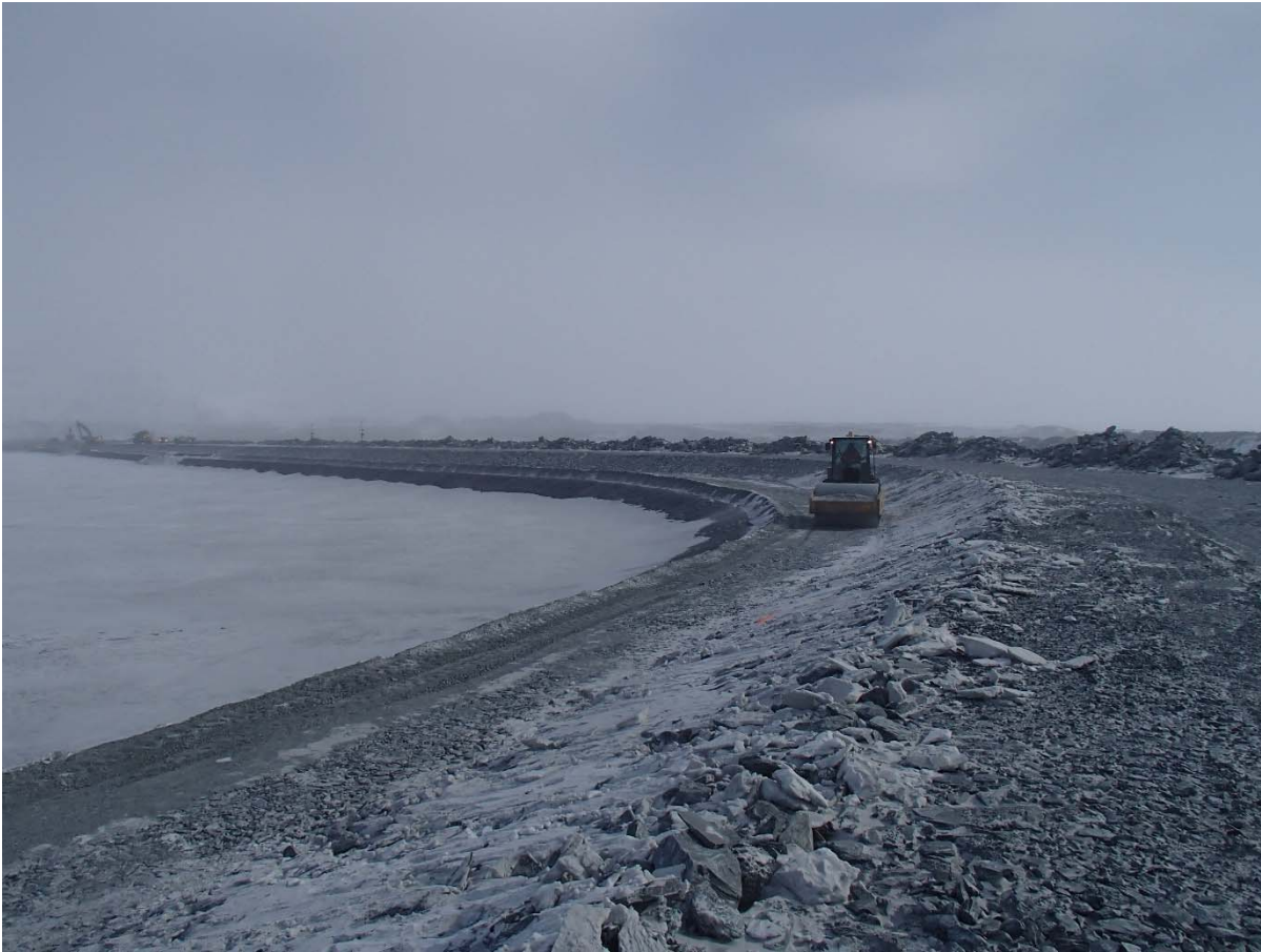
Photograph CD-1831: From Sta. 40+730/-24 m, looking NE. Compaction of the first 0.5 m lift (approx.) of fine and coarse filters material at El. 143.5 m with a 10-tonne smooth-drum compactor with vibration (6 passes) from Sta. 40+730 m to 0+830 m and from Sta. 0+175 m to 0+490 m.
