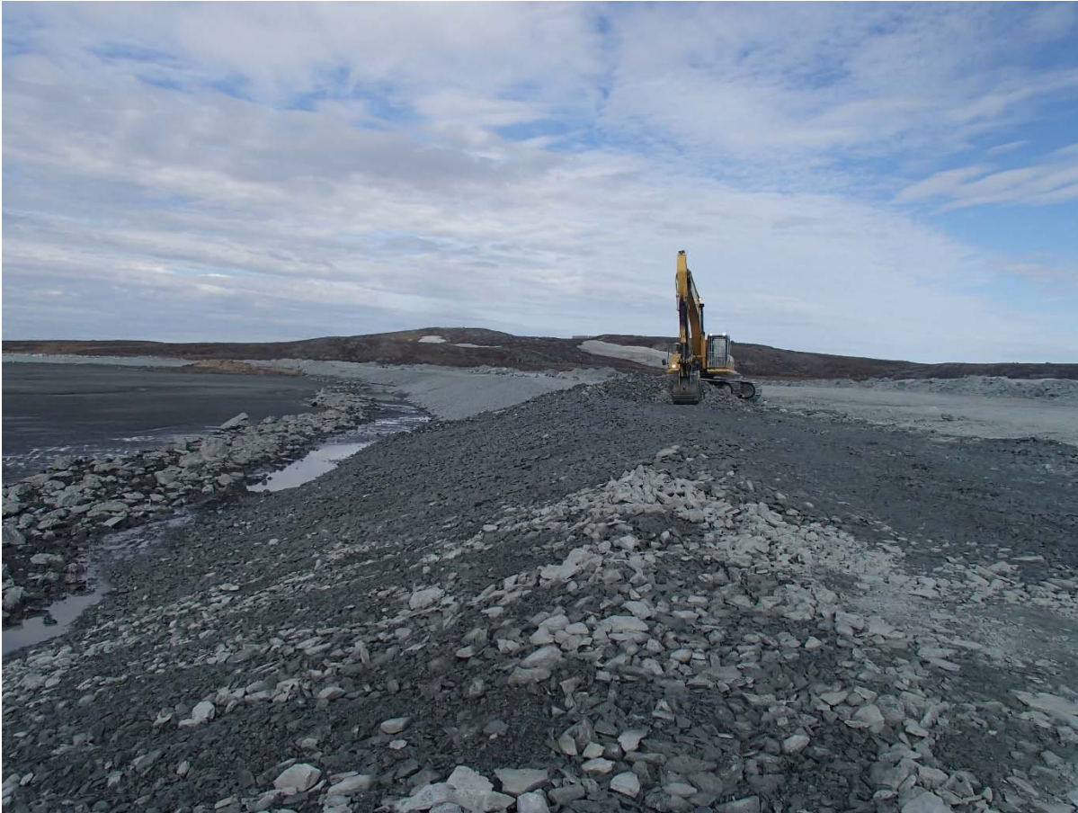
Photograph NCIS-030: From Sta. 2+140/-29 m (approx.), looking W. Placement of a 0.5 m thick lift of coarse filter in the upstream slope from El. 150 m to 152 m with an excavator from Sta. 2+105 m to 1+930 m. Notice the presence of water ponding at the bottom of the slope.
