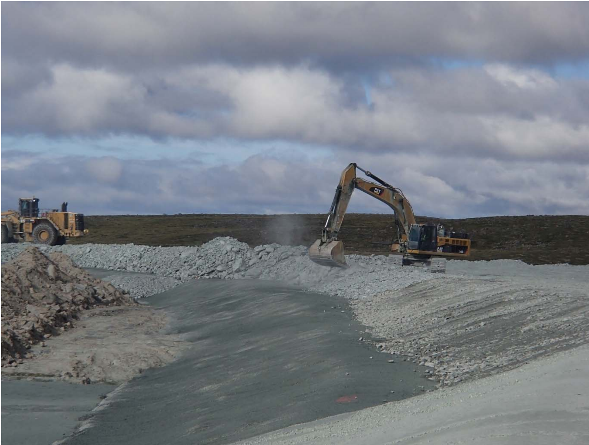
Photograph NCIS-132: From Sta. 1+940/-20 m (approx.), looking W. Profiling of the upstream slope (3H:1V) from El. 152 to 154 m with an excavator from Sta. 1+780 m to 1+660 m.
