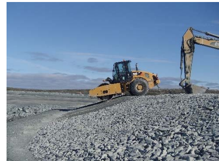
NCIS-105 (2018-07-21), looking NW from Sta. 2+630/-34 m (approx.). Compaction of the 0.5 m lift (approx.) of coarse filter between El. 152 m and 154 m with a 10-tonne smooth-drum compactor with vibration (4 passes) in the upstream slope from Sta. 2+710 m to 2+411 m.
