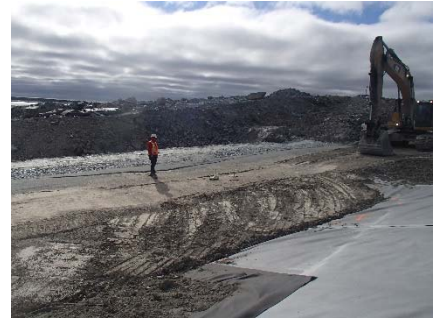
SD3-334 (2018-07-13), looking SE from Sta. 20+780/-26 m. Compaction of the second 0.5 m thick lift of compacted sieved till and third lift of fine filter, coarse filter and fine rockfill of the upstream toe liner tie-in with a 10 tonne smooth-drum compactor with vibrations from Sta. 20+770 m to 20+800 m.
