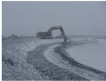
CD-1827 (2018-05-06), looking SW from Sta. 0+940/-16 m. Placement of a 0.5 m thick lift of fine filter from El. 143 m to 143.5 m with an excavator from Sta. 40+730 m to 0+835 m.
