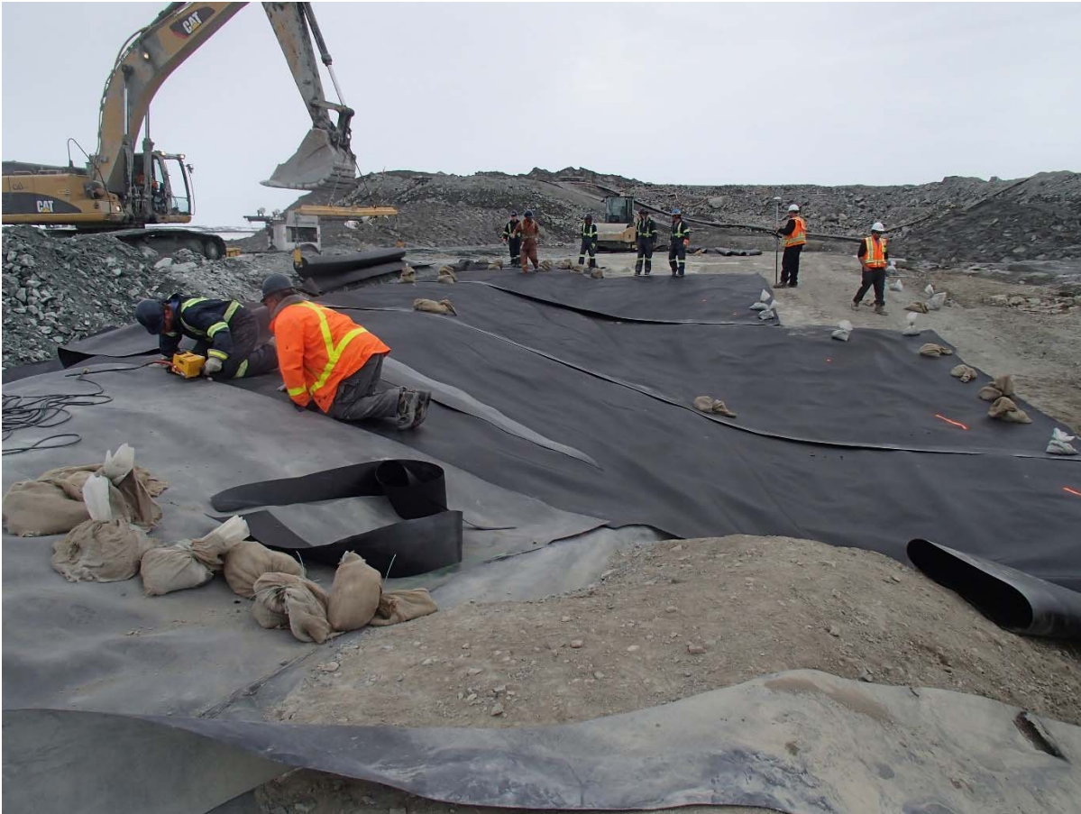
Photograph SD3-315: From Sta. 20+615/-46 m, looking W. Installation of the geotextile on the upstream slope 3H:1V between El. 143 m and 145 m from Sta. 20+593 m to 20+610 m and installation of the LLDPE liner on the upstream slope 3H:1V between El. 143 m and 145 m from Sta. 20+593 m to 20+610 m (panel numbers 965 to 967).
