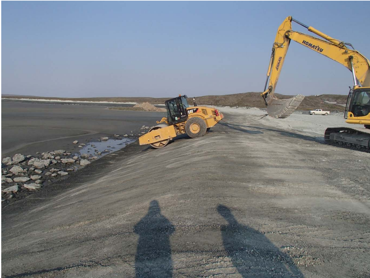
Photograph NCIS-088: From Sta 2+000/-35 m (approx.), looking W. Compaction of the 0.5 m lift (approx.) of fine filter between El. 150 m and 152 m with a 10-tonne smooth-drum compactor (4 passes) in the upstream slope from Sta. 2+028 m to 1+650 m.
