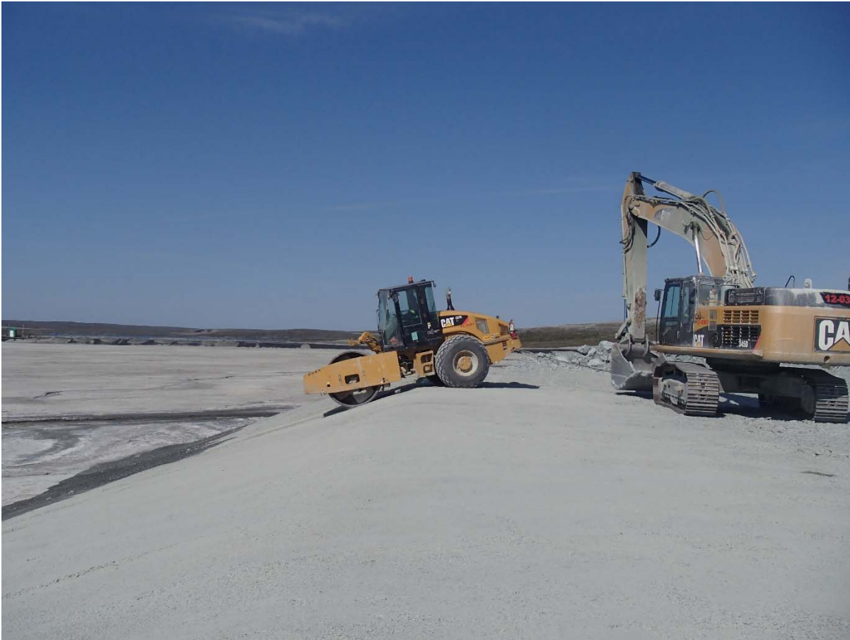
Photograph NCIS-126: From Sta. 1+140/-98 m (approx.), looking W. Compaction of the 0.5 m lift (approx.) of coarse filter between El. 150 m and 152 m with a 10-tonne smooth-drum compactor with vibration (4 passes) in the upstream slope from Sta. 1+240 m to 1+100 m.
