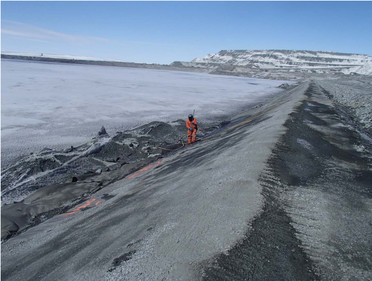
Photograph CD-1586: From Sta. 0+670/-24 m, looking N. Clean-up of the fine filter placed against the slope at the deposition finger at approx. Sta. 0+670 m with pressurized air stream to expose 1 m of LLDPE liner, in preparation for the new liner installation.
