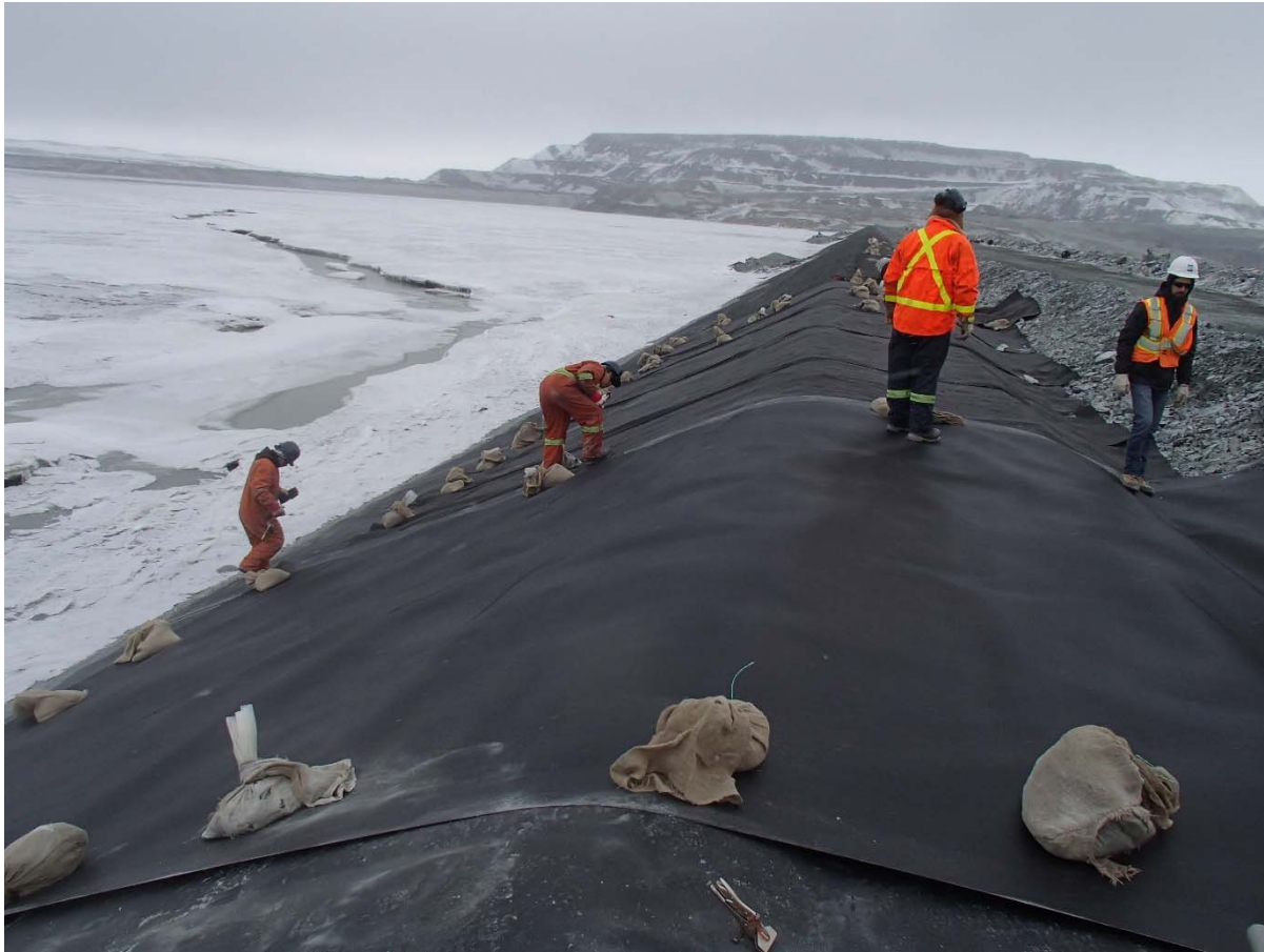
Photograph CD-1874: From Sta. 0+760/-26 m, looking N. Installation of the geotextile on the upstream slope 2H:1V between El. 143 m and 145 m from Sta. 0+760 m to 0+740 m.
