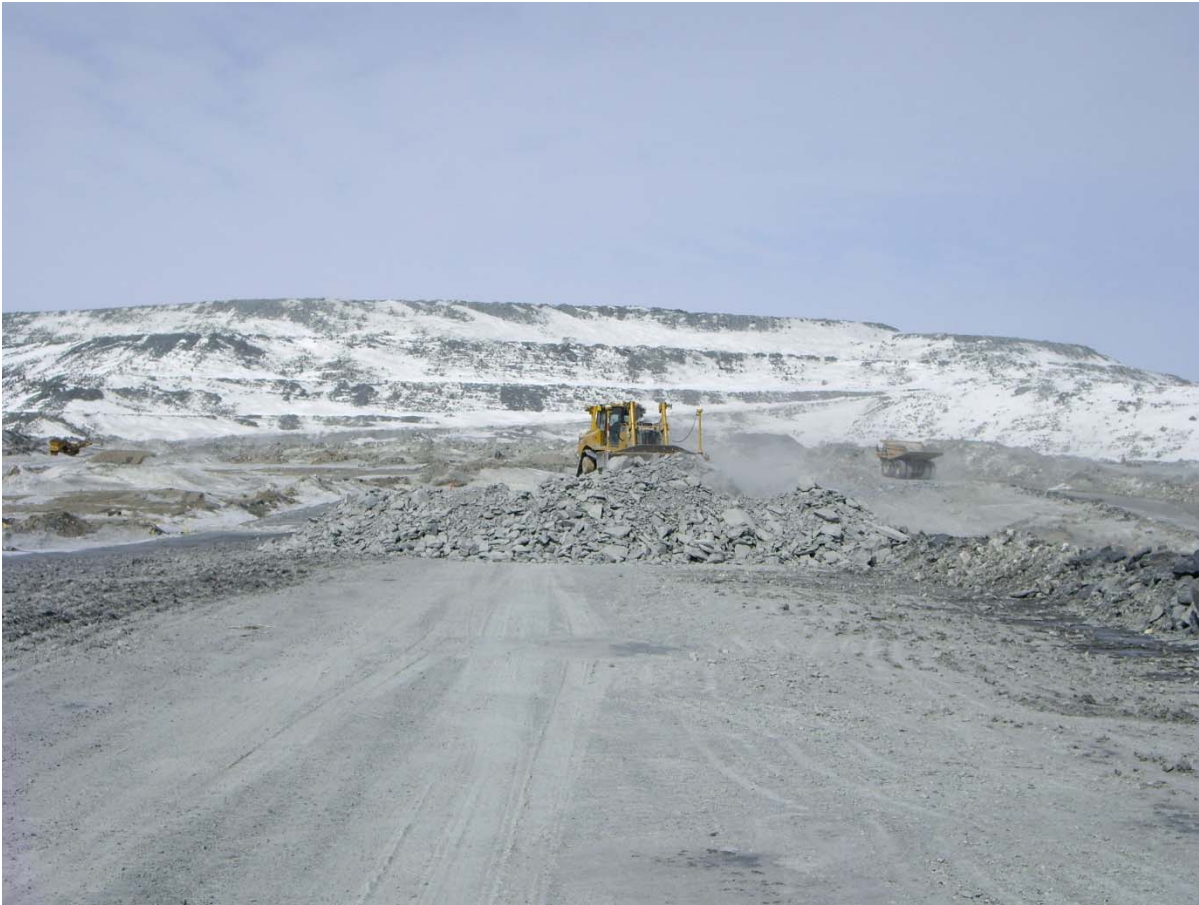
Photograph CD-1797: From Sta. 0+320/-20 m looking N. Placement a 2 m thick (approx.) lift of volcanic rockfill from El. 143 m to El. 145 m from 0+250 to 0+400 m (o.s. -28 to -18 m).
