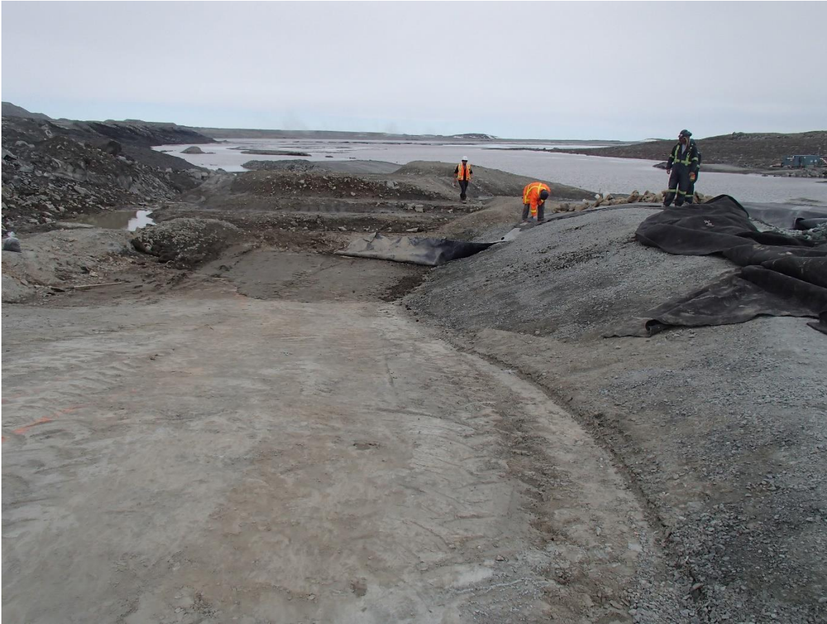
Photograph SD3-314: From Sta. 20+590/-32 m, looking E. View of the liner bedding ready for geosynthetics installation.
