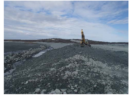
NCIS-030 (2018-06-20), looking W from Sta. 2+140/-29 m. Placement of a 0.5 m thick lift of coarse filter in the upstream slope from El. 150 m to 152 m with an excavator from Sta. 2+105 m to 1+930 m. Notice the presence of water ponding at the bottom of the slope.
