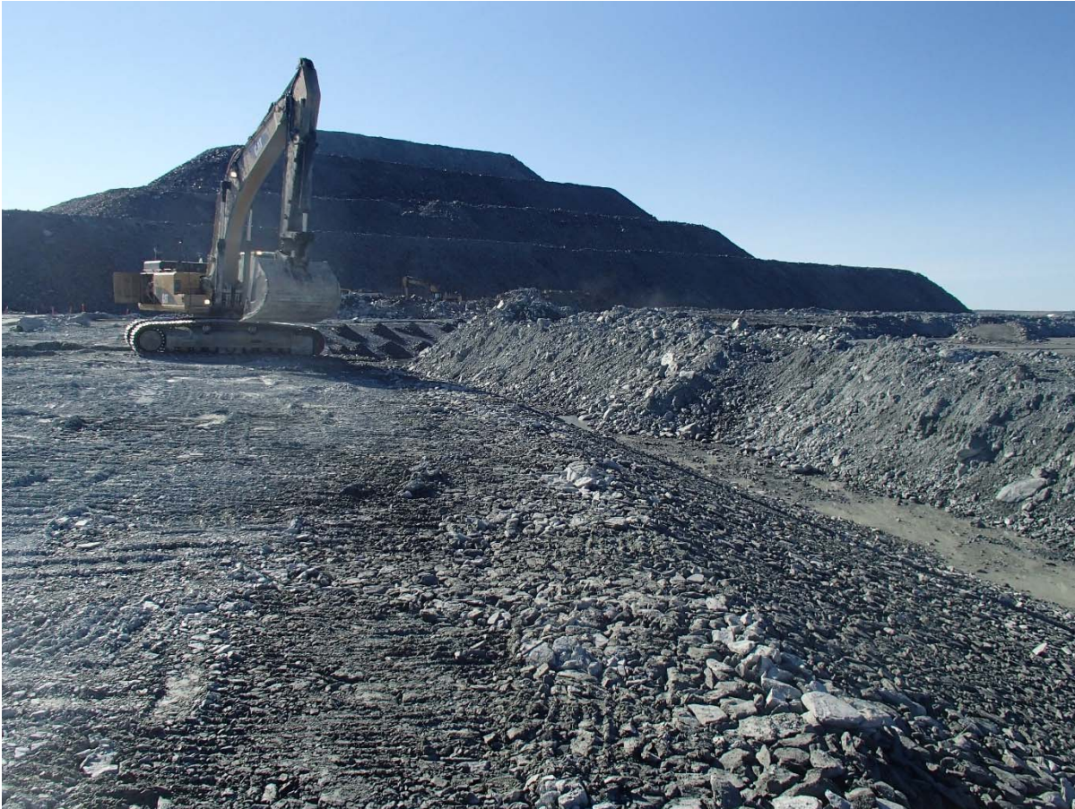
Photograph NCIS-051: From Sta. 2+630/-34 m (approx.), looking SE. Placement of a 0.5 m thick lift of coarse filter in the upstream slope from El. 150 m to 152 m with an excavator from Sta. 2+640 m to 2+815 m.
