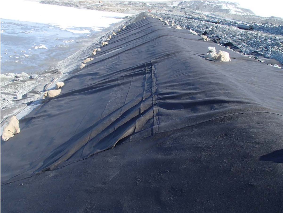
Photograph CD-1881: From Sta. 0+530/-27 m, looking N. View of a geotextile panel with a horizontal weld in the slope at Sta. 0+520 m before its removal.
