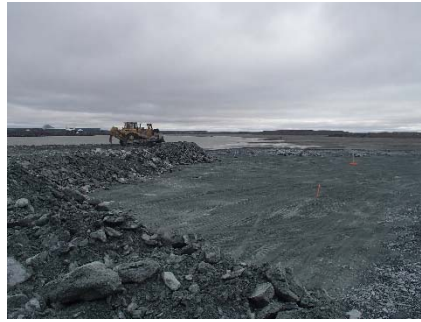
NCIS-083 (2018-07-07), looking SW from Sta. 1+140/52 m. Placement of a 2 m thick (approx.) lift of IV rockfill from El. 150 m to El. 152 m (approx.) with a dozer from Sta. 1+160 m to 1+170 m (-64 m to -111 m).
