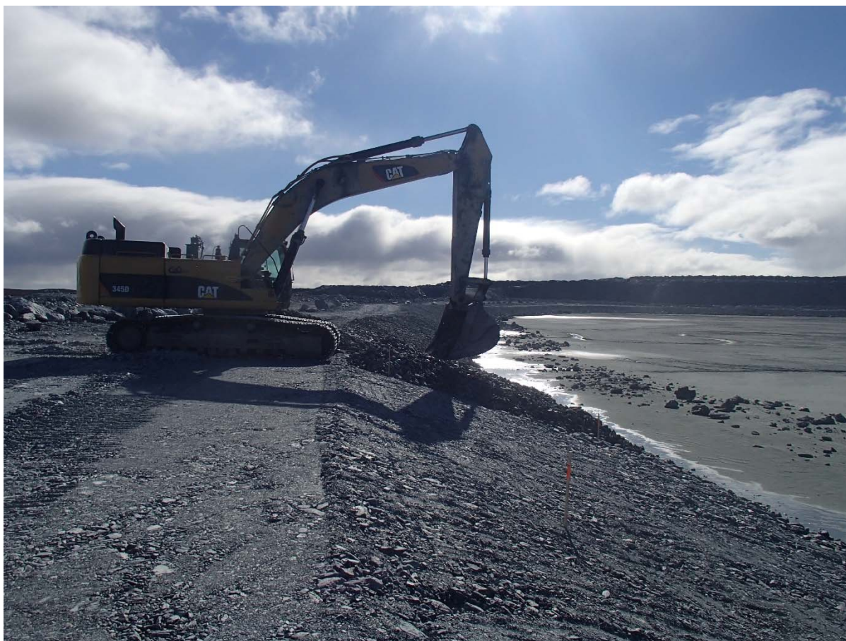
Photograph NCIS-033: From Sta. 1+900/-21 m (approx.), looking E. Placement of a 0.5 m thick lift of coarse filter in the upstream slope from El. 150 m to 152 m with an excavator from Sta. 1+930 m to 1+715 m.
