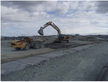
SD3-350 (2018-07-18), looking SE from Sta. 20+740/-24 m. Placement of a 0.5 m thick lift of coarse filter on the top of 0.5 m lift of low quality till (0-150 mm) the fine filter on the upstream toe liner with an excavator from Sta. 20+777 m to 20+807 m.
