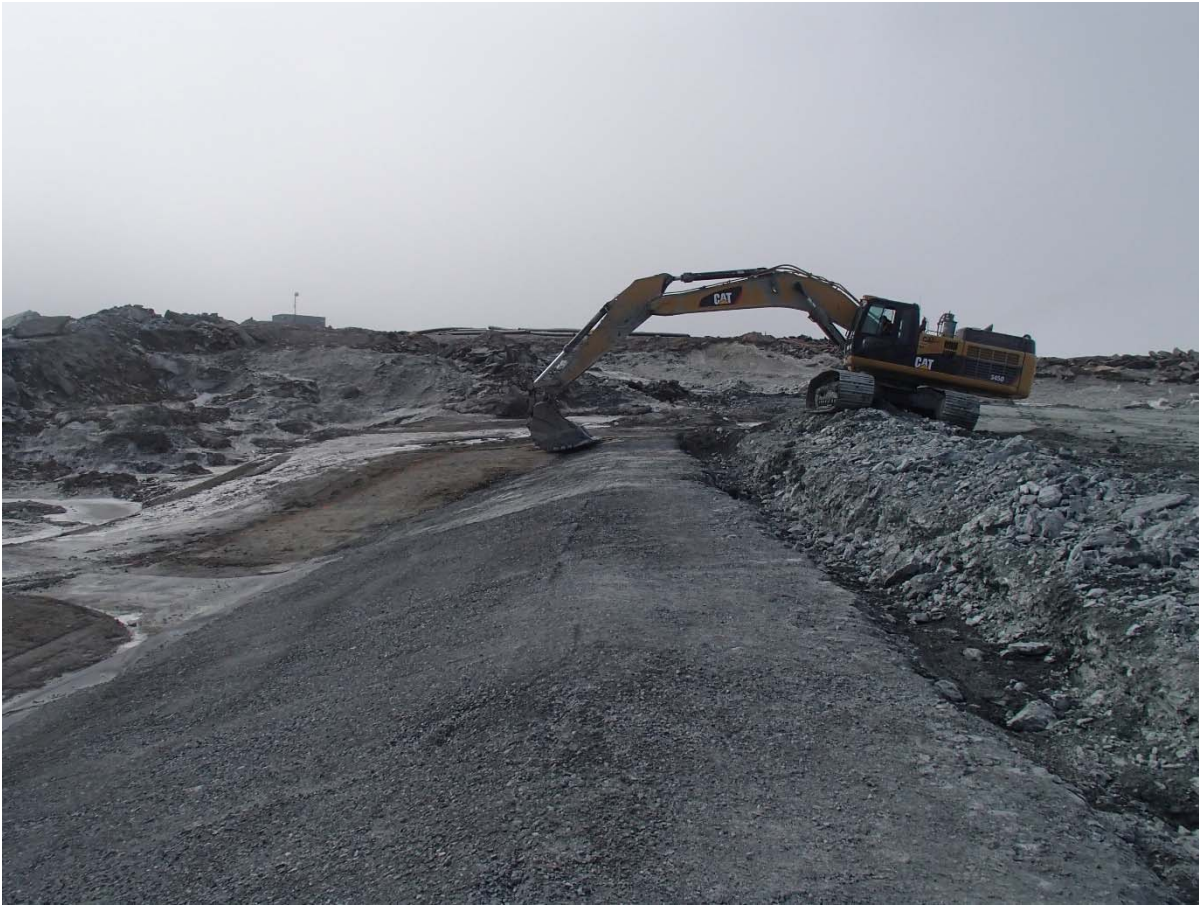
Photograph SD3-306: From Sta. 20+780/-25 m, looking S. Correction of the surface of the fine filter in the upstream slope and the top of the first class compacted sieved till layer with an excavator from Sta. 20+803 m to 20+793 m.
