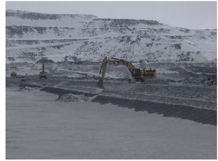
CD-1834 (2018-05-08), looking NE from Sta. 40+760/-23 m. Placement of a first 0.5 m thick lift of coarse filter from El. 143 m to 143.5 m on length of approx. 5 m with an excavator at the location of the deposition finger at Sta 0+520 m and 0+660 m.
