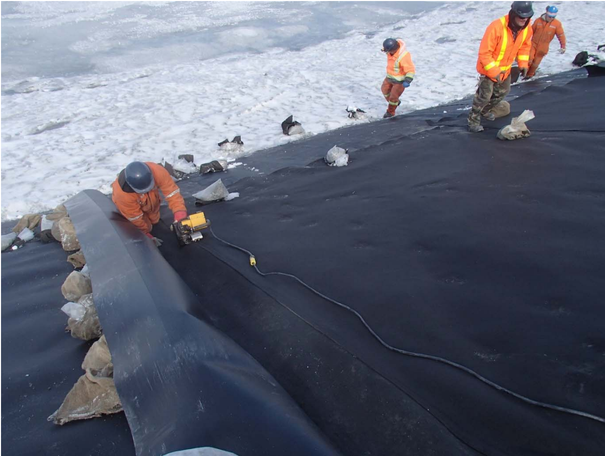
Photograph CD-1869: From Sta. 0+915/-30 m, looking W. Installation of the geotextile on the upstream slope 2H:1V between El. 143 m and 145 m from Sta. 0+935 m to 0+900 m.
