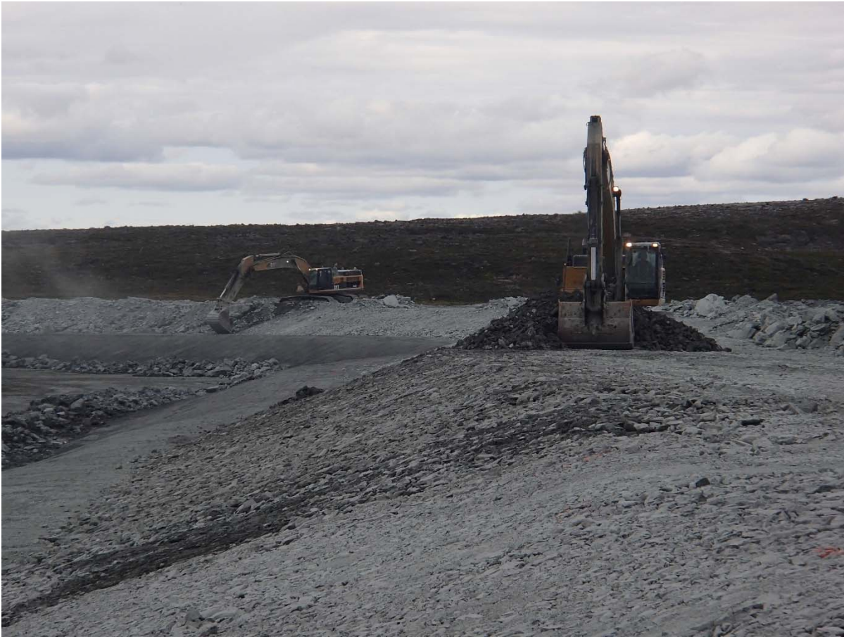
Photograph NCIS-109: From Sta. 2+450/-21 m (approx.), looking N. Placement of a 0.5 m thick lift of coarse filter in the upstream slope from El. 152 m to 154 m with an excavator from Sta. 2+293 m to 2+411 m.
