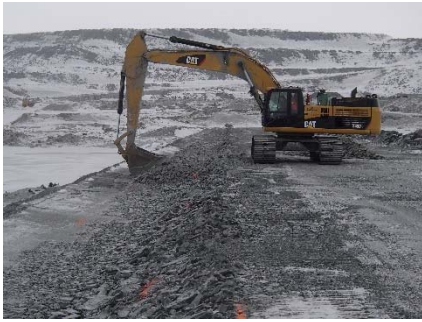
CD-1841 (2018-05-10), looking N from Sta. 0+475/-14 m. Placement of a third 0.5 m thick lift of coarse filter from El. 144 m to 144.5 m with an excavator from Sta. 0+335 m to 40+730 m.
