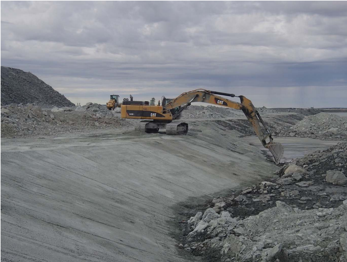
Photograph NCIS-078: From Sta. 2+760/-39 m (approx.), looking S. Placement of a 0.5 m thick lift of fine filter over the coarse filter in the upstream slope from El. 150 m to 152 m with an excavator from Sta. 2+800 m to 2+980 m.
