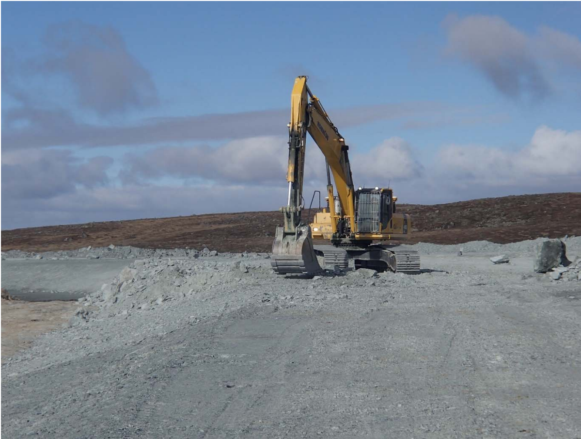
Photograph NCIS-034: From Sta. 1+900/-21 m (approx.), looking W. Profiling of the upstream slope (3H:1V) from El. 150 to 152 m with an excavator from Sta. 1+860 m to 1+750 m.
