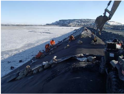
CD-1871 (2018-05-28), looking N from Sta. 0+910/-25 m. Installation of the geotextile on the upstream slope 2H:1V between El. 143 m and 145 m from Sta. 0+900 m to 0+870 m.
