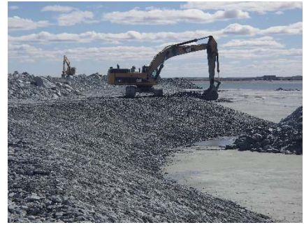
NCIS-075 (2018-07-03), looking S from Sta. 2+860/-36 m. Placement of a 0.5 m thick lift of coarse filter in the upstream slope from El. 150 m to 152 m with an excavator from Sta. 2+815 m to 2+980 m.
