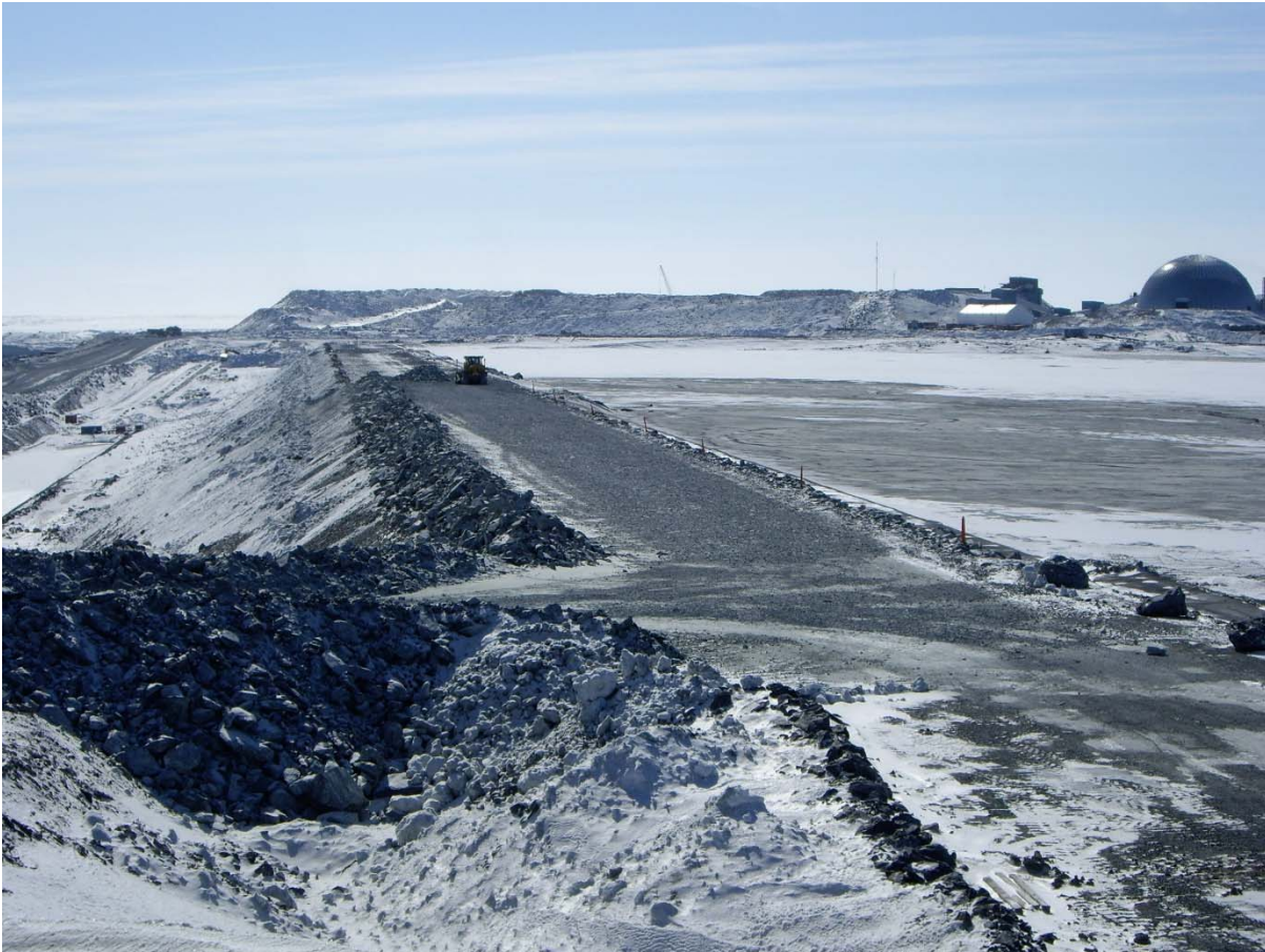
Photograph CD-1799: From Sta. 0+080/-25 m looking S. Placement of a 2 m thick (approx.) lift of intermediate volcanic (IV) rockfill from El. 143 m to El. 145 m from 0+340 to 0+435 m (o.s. -28 to -18 m).
