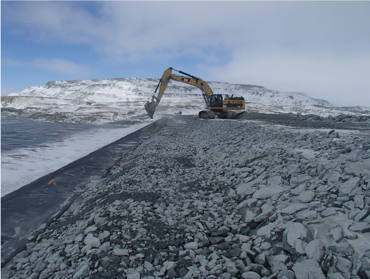
Photograph CD-1829: From Sta 0+410/-22 m, looking N. Placement of a 0.5 m thick lift of coarse filter from El. 143 m to 143.5 m with an excavator from Sta. 0+170 m to 0+460 m and placement of a 0.5 m thick lift of fine filter from Sta. 0+170 m to 0+380 m.
