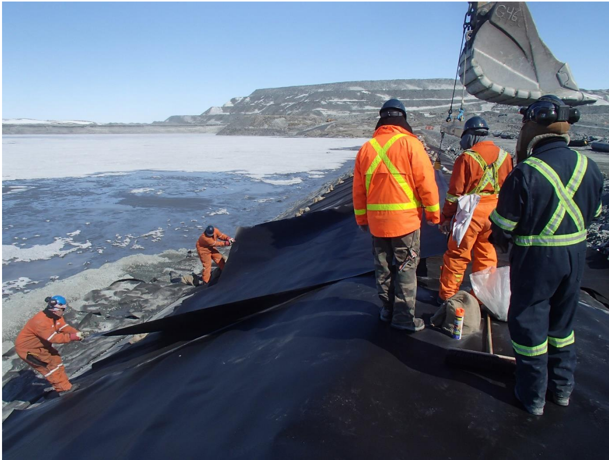
Photograph CD-1883: From Sta. 0+525/-26 m, looking N. Installation of the LLDPE liner on the upstream slope 2H:1V between El. 143 m and 145 m from Sta. 0+610 m to 0+480 m (panel numbers 868 to 886).
