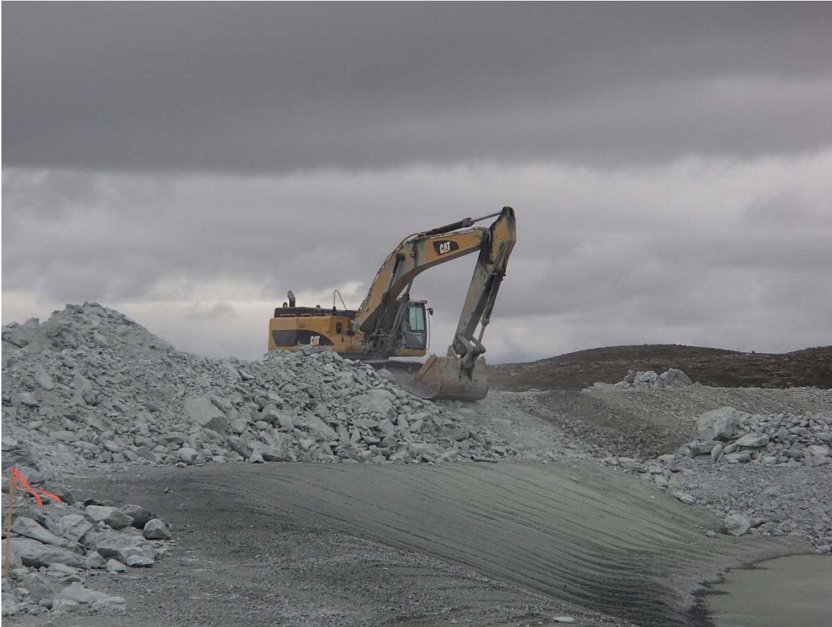
Photograph NCIS-134: From Sta. 1+630/-32 m (approx.), looking NE. Completion of the profiling of the upstream slope (3H:1V) from El. 152 to 154 m with an excavator from Sta. 1+700 m to 1+660 m.
