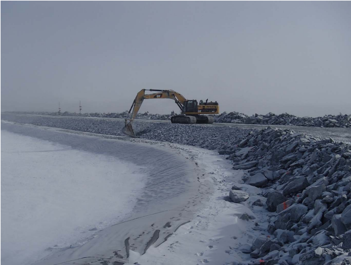
Photograph CD-1824: From Sta 40+760/-25 m, looking NE. Profiling of the upstream slope (2H:1V) from El. 143 to 145 m with an excavator between Sta. 0+830 m and 40+730 m.
