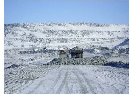
CD-1798 (2018-04-24), looking N from Sta. 0+500/-15 m. Placement a 2 m thick (approx.) lift of intermediate volcanic rockfill from El. 143 m to El. 145 m from 0+340 to 0+435 m (o.s. -28 to -18 m).
