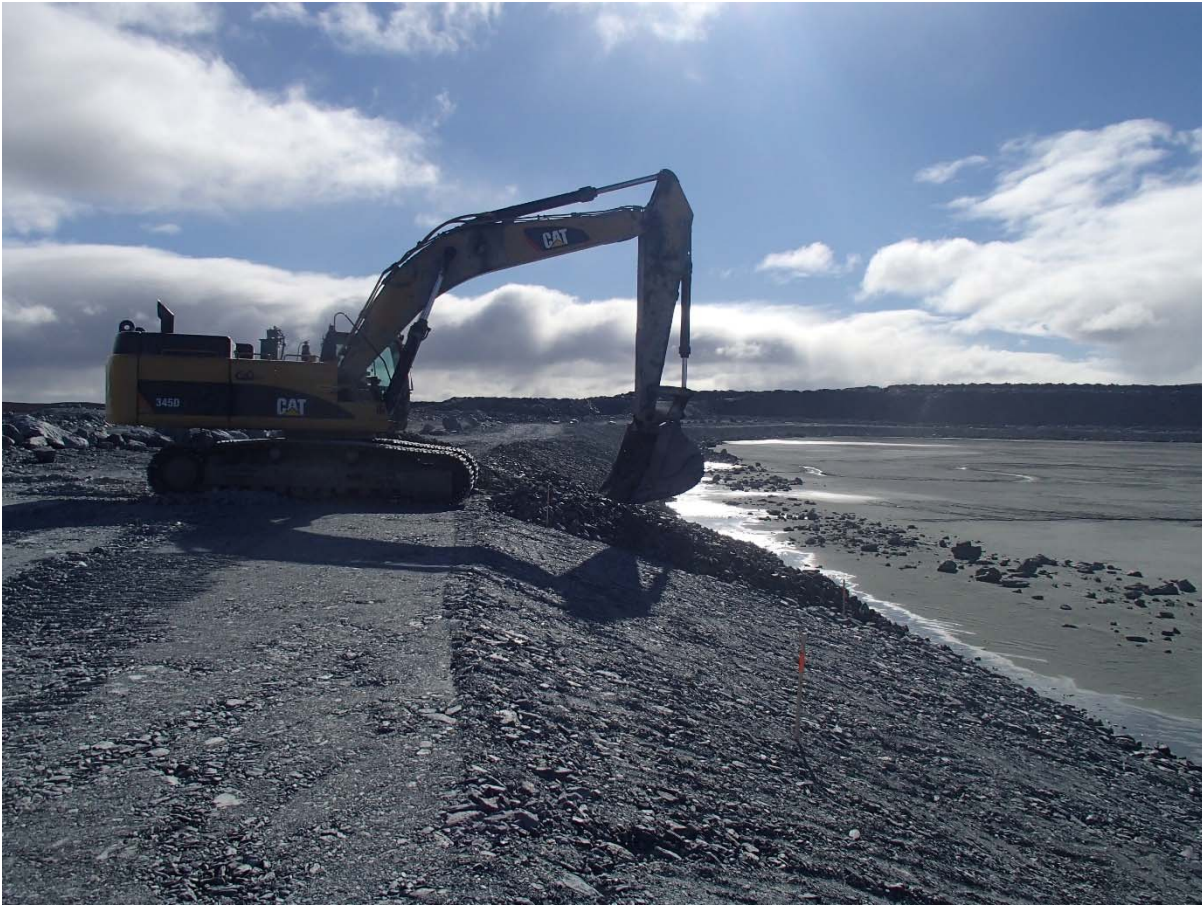
Photograph NCIS-033: From Sta. 1+900/-21 m (approx.), looking E. Placement of a 0.5 m thick lift of coarse filter in the upstream slope from El. 150 m to 152 m with an excavator from Sta. 1+930 m to 1+715 m.
