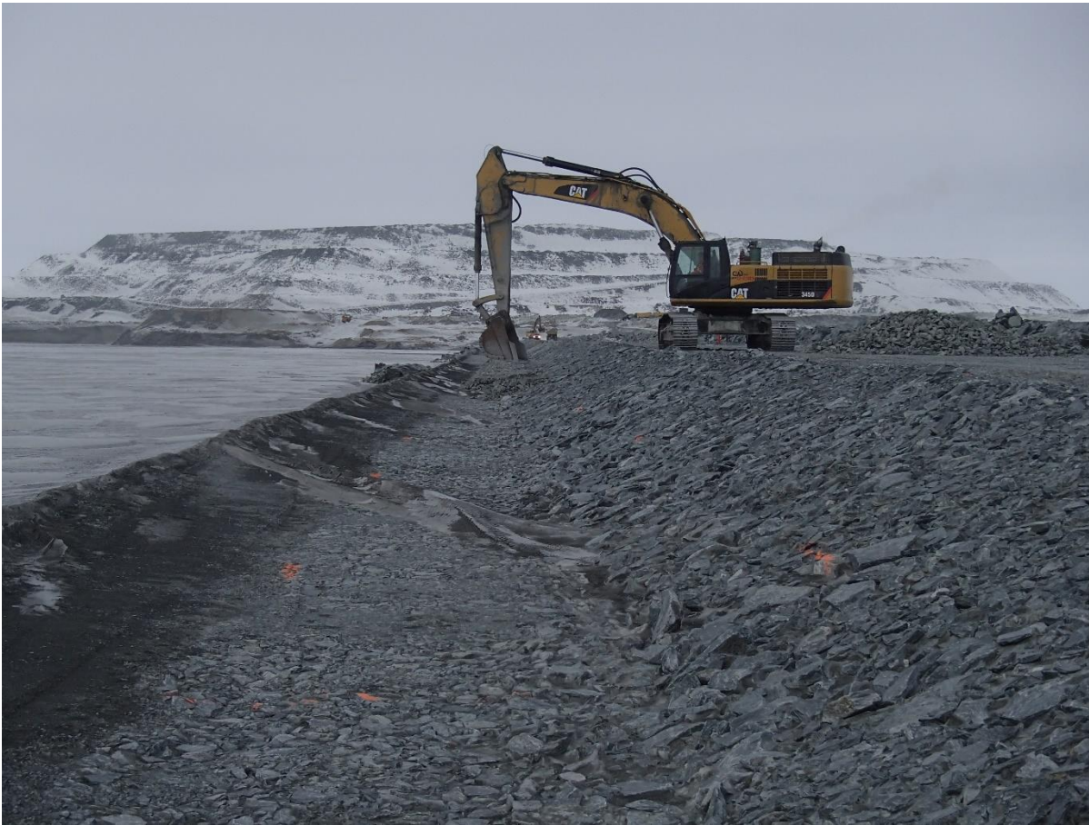
Photograph CD-1837: From Sta 0+940/-25m, looking N. Placement of a second 0.5 m thick lift of coarse filter from El. 143.5 m to 144 m with an excavator from Sta. 0+290 to 0+500 m and from Sta. 0+835 to 0+930 m.
