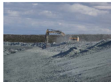
NCIS-108 (2018-07-22), looking N from Sta. 2+490/-32 m (approx.). Profiling of the upstream slope (3H:1V) from El. 152 to 154 m with an excavator from Sta. 2+159 m to 2+409 m.
