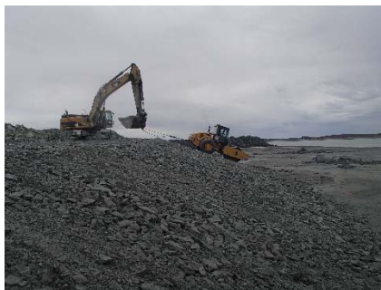
NCIS-080 (2018-07-05), looking S from Sta. 2+800/-38 m. Compaction of the 0.5 m lift (approx.) of coarse filter between El. 150 and 152 m with a 10-tonne smooth-drum compactor (4 passes) in the upstream slope from Sta. 2+925 m to 3+160 m and from Sta. 1+300 m to 1+200 m.
