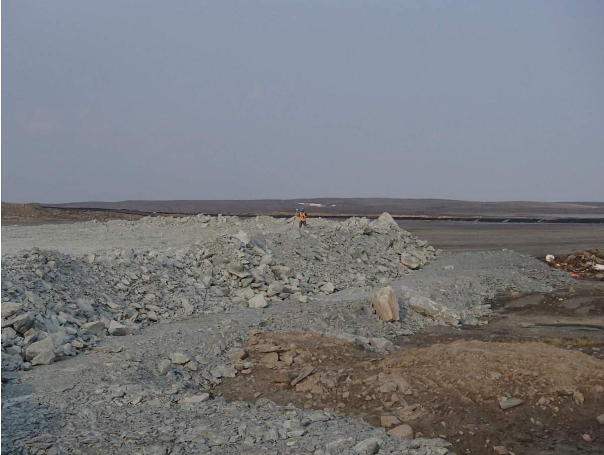
Photograph NCIS-085: From Sta 1+150/-67m (approx.), looking SW. Placement of a 2 m thick (approx.) lift of UM rockfill from El. 150 m to El. 152 m (approx.) with a dozer from Sta. 1+130 m to 1+100 m (-55 m to -78 m).
