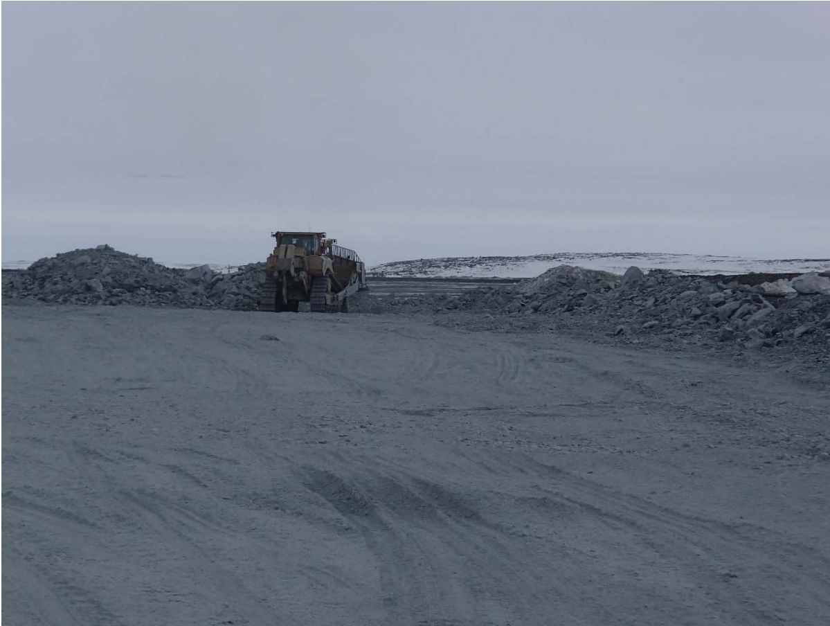
Photograph NCIS-021: From Sta. 1+550 m (approx.), looking S. Placement a 2 m thick (approx.) lift of UM rockfill from El. 150 m to El. 152 m (approx.) with a dozer from Sta. 1+535 m to 1+500 m (offset unavailable).
