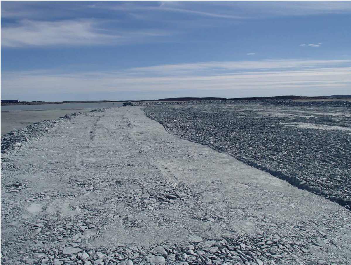
Photograph NCIS-050: From Sta. 1+230/-55 m (approx.), looking S. Compaction of the 1.5 to 2 m lift (approx.) of ultramafic (UM) rockfill at El. 150 m with a 10-tonne smooth-drum compactor with vibration (6 passes) between the haul truck traffic lane and the upstream slope from Sta. 1+220 to 1+130 m (offset -91 to -44 m).
