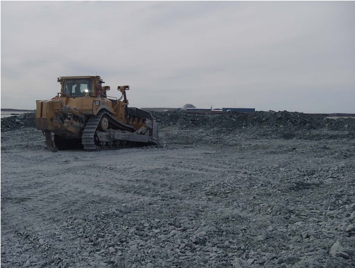
Photograph NCIS-041: From Sta. 1+220/-7 m (approx.), looking S. Placement of a 1.5 to 2 m thick (approx.) lift of UM rockfill from El. 148 m to El. 150 m (approx.) with a dozer from Sta. 1+197 m to 1+150 m (-7 m to -41 m).
