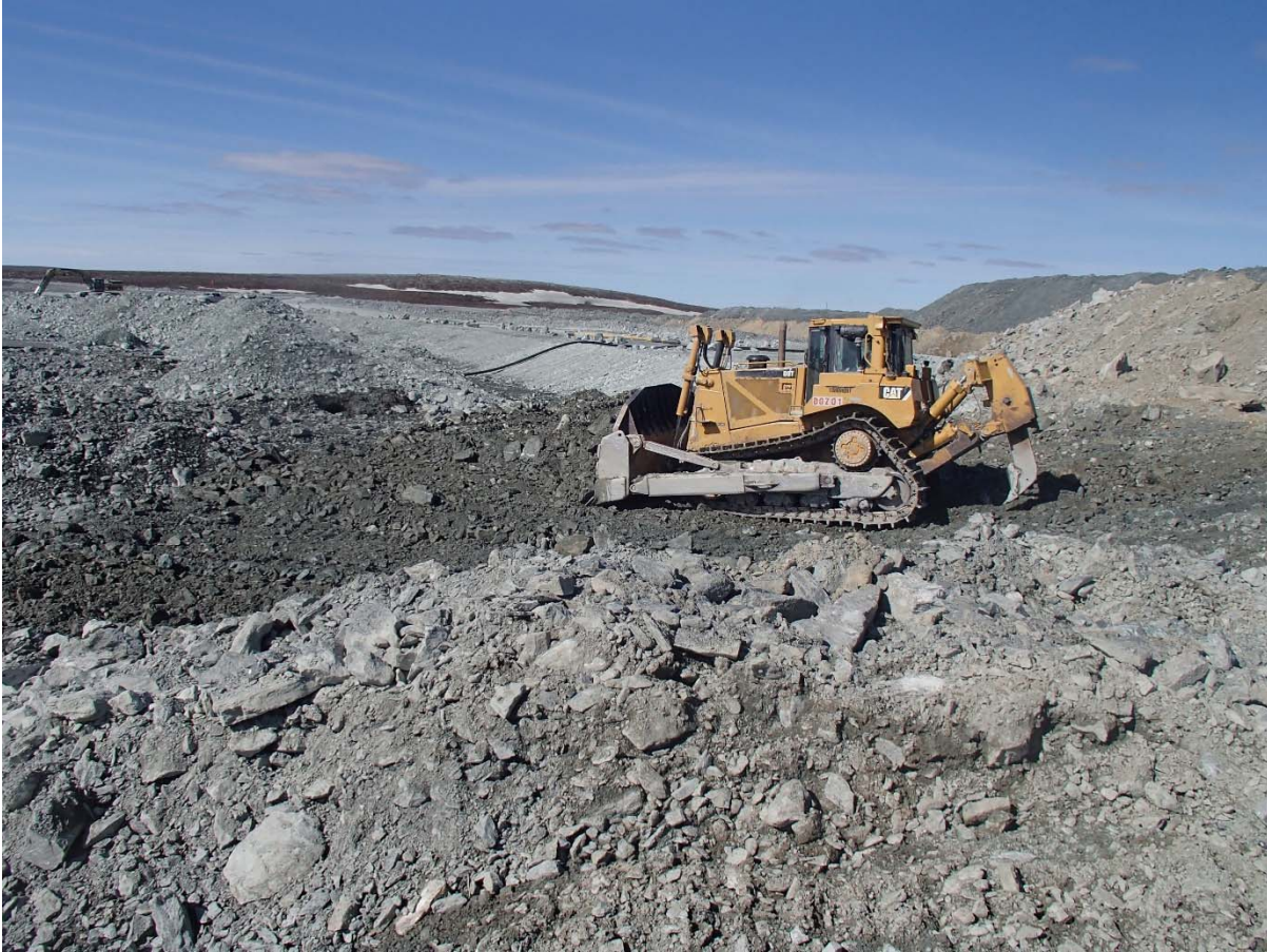
Photograph NCIS-049: From Sta. 2+870/-28 m (approx.), looking N. Removing of UM rockfill material from the capping with a dozer to level the surface to El. 150 m from Sta. 2+760 m to 2+850 m (o.s. -29 to -17 m).
