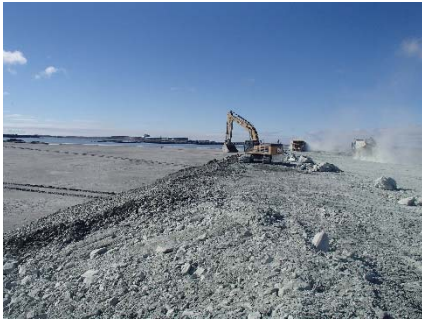
NCIS-058 (2018-06-29), looking S from Sta. 1+340/-34 m. Placement of a 0.5 m thick lift of coarse filter in the upstream slope from El. 148 m to 152 m with an excavator from Sta. 1+340 m to 1+270 m.
