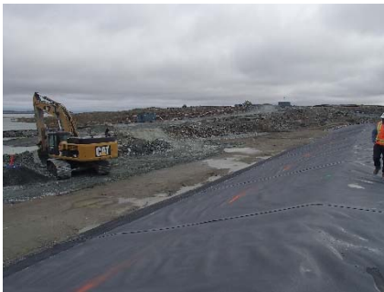
SD3-318 (2018-07-07), looking SE from Sta. 20+710/-24 m. Placement of IV rockfill in the water up to El. 142m with an excavator from Sta. 20+785 m to 20+730 m, at the bottom of the upstream slope of SD3 to widen the rockfill layer and allow access to the erosion protection.
