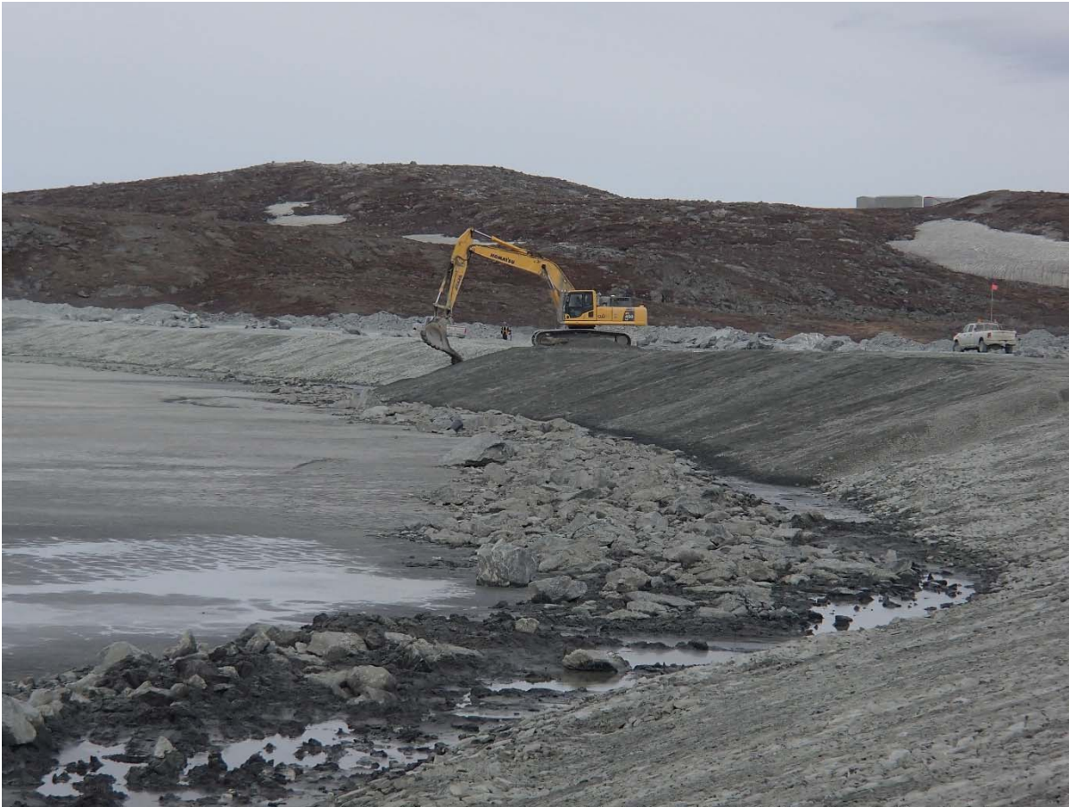
Photograph NCIS-040: From Sta. 2+185/-25 m (approx.), looking W. Placement of a 0.5 m thick lift of fine filter over the coarse filter in the upstream slope from El. 150 m to 152 m with an excavator from Sta. 2+305 m to 2+460 m and from Sta. 1+980 m to 1+835 m.
