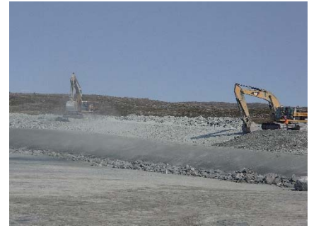
NCIS-111 (2018-07-23), looking NW from Sta. 2+320/-22 m (approx.). Profiling of the upstream slope (3H:1V) from El. 152 to 154 m with an excavator from Sta. 2+159 m to 2+000 m and placement of a 0.5 m thick lift of coarse filter in the upstream slope from El. 152 m to 154 m with an excavator from Sta. 2+293 m to 2+080 m.
