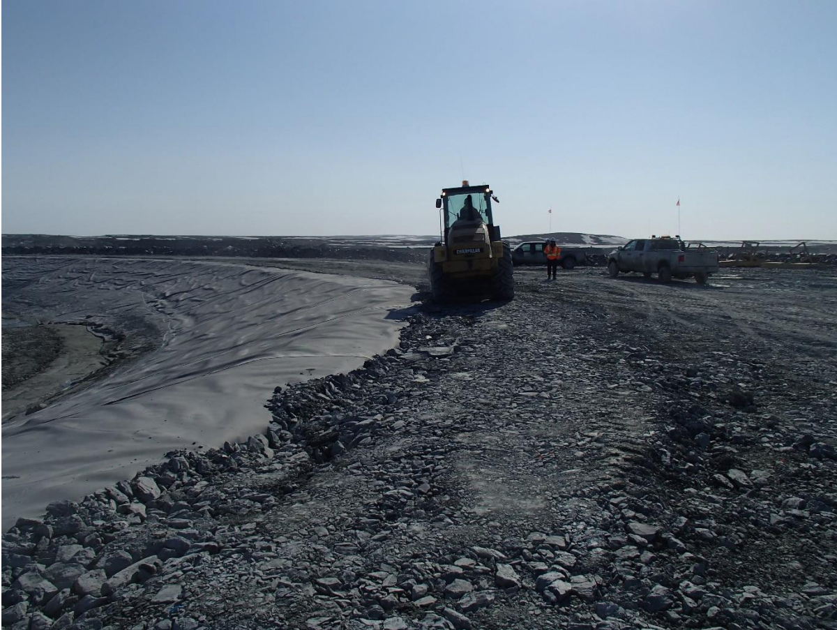
Photograph CD-1895: From Sta. 40+670/-15 m, looking E. Compaction of the geosynthetics tie-in material at El. 145 m with a 10-tonne smooth-drum compactor with vibration (4 passes) from Sta. 40+670 m to 0+950 m (approx.).
