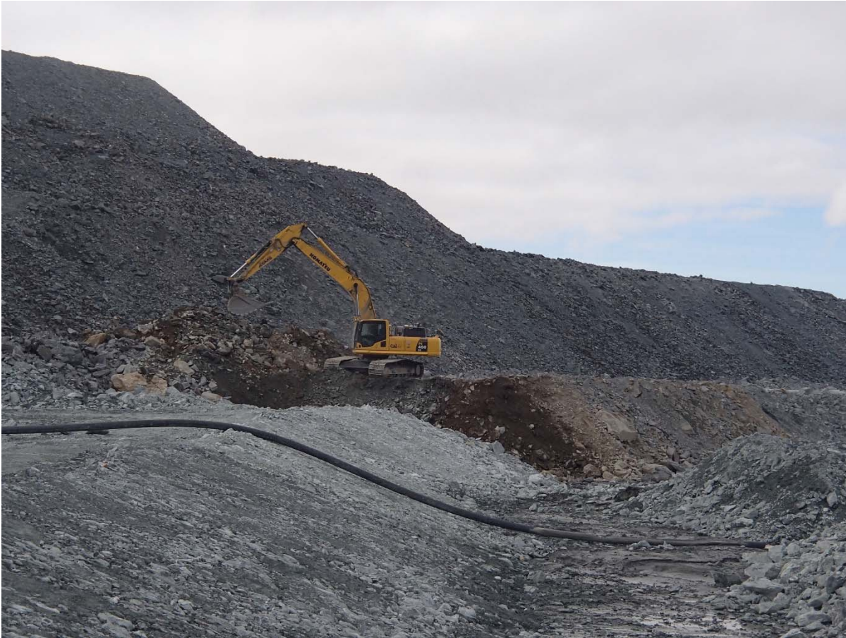
Photograph NCIS-046: From Sta. 2+680/-18 m (approx.), looking SE. Removal of till material mixed with the UM rockfill of the capping (about 1 to 2 m thick along the slope) with an excavator from Sta. 2+760 m to 2+850 m (o.s. -35 to -17 m).
