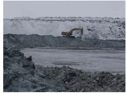
NCIS-012 (2018-05-22), looking NW from Sta. 2+000 m. Profiling of the upstream slope (3H:1V) from El. 150 to 152 m with an excavator from Sta. 2+325 m to 2+275 m (approx.).
