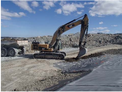
SD3-332 (2018-07-12), looking SE from Sta. 20+775/-23 m. Placement of a first 0.5 m thick lift of compacted sieved till over the LLDPE geomembrane on the upstream toe liner tie-in with an excavator from Sta. 20+775 m to 20+800 m.
