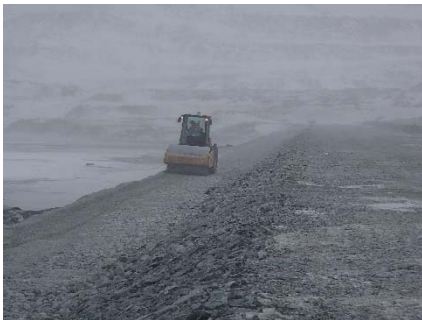
CD-1835 (2018-05-08), looking N from Sta. 0+830/-20 m. Compaction of the first 0.5 m lift (approx.) of fine and coarse filters material at El. 143.5 m with a 10-tonne smooth-drum compactor with vibration (6 passes) from Sta 0+490 m to 0+835 m.
