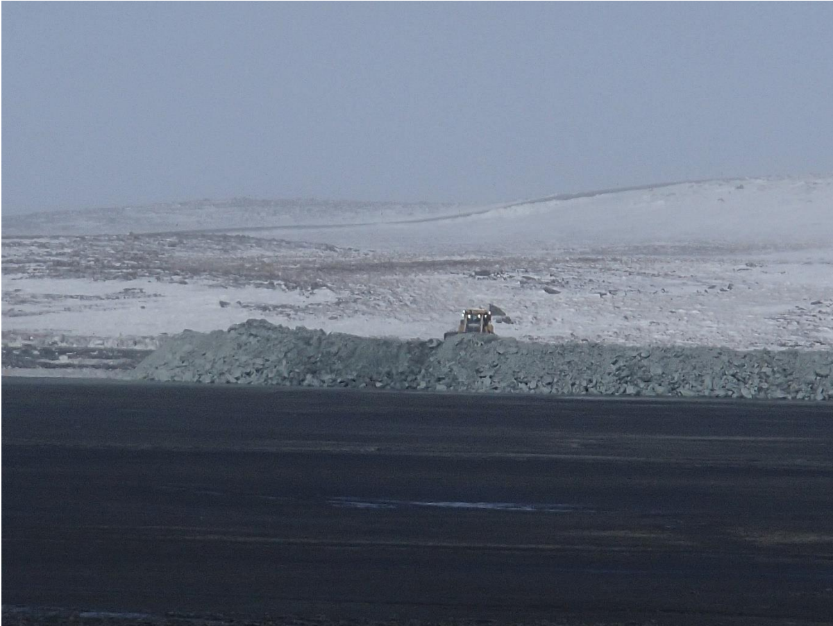
Photograph NCIS-023: From Sta. 2+570 m (approx.), looking W. Placement of a 2 m thick (approx.) lift of UM rockfill from El. 150 m to El. 152 m (approx.) with a dozer from Sta. 1+500 m to 1+450 m (o.s. unavailable). The material is of good quality and is well graded.
