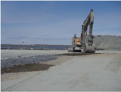
SD3-353 (2018-07-22), looking SW from Sta. 20+580/-49 m. View of SD3 at the end of the 2018 construction phase.
