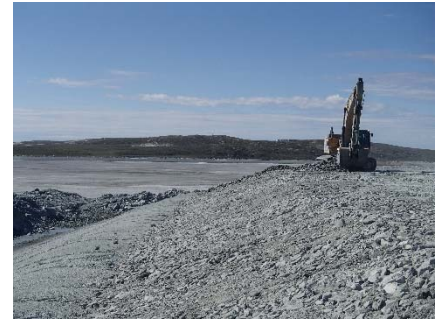
NCIS-102 (2018-07-20), looking W from Sta. 2+680/-21 m (approx.). Placement of a 0.5 m thick lift of coarse filter in the upstream slope from El. 152 m to 154 m with an excavator from Sta. 2+575 m to 2+710 m and from Sta. 2+411 m to 2+460 m.
