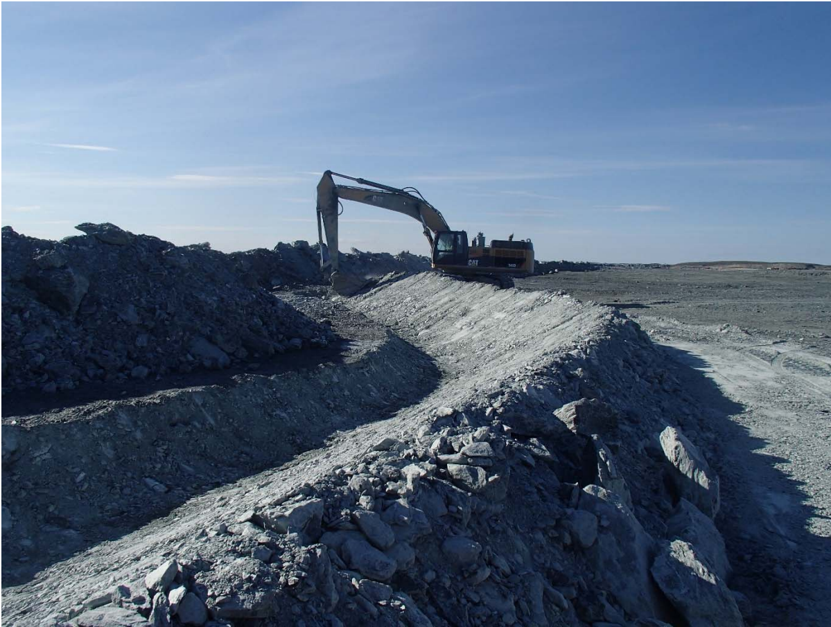
Photograph NCIS-116: From Sta. 1+700/+37 m (approx.), looking SE. Excavation of a 0.8 m (approx.) deep, 1 m wide shallow ditch in the rockfill capping with an excavator from Sta. 1+500 m to 1+455 m.
