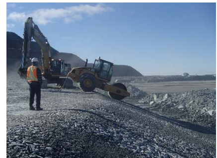
NCIS-054 (2018-06-28), looking SE from Sta. 2+580/-31 m. Compaction of the 0.5 m lift (approx.) of coarse filter between El. 150 and 152 m with a 10-tonne smooth-drum compactor with vibration (4 passes) in the upstream slope from Sta. 2+560 m to 2+815 m.
