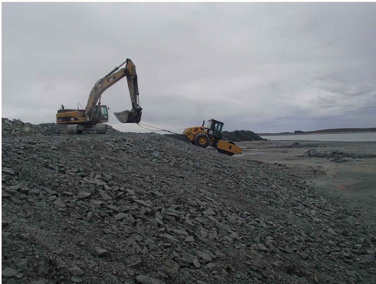
Photograph NCIS-080: From Sta. 2+800/-38 m (approx.), looking S. Compaction of the 0.5 m lift (approx.) of coarse filter between El. 150 and 152 m with a 10-tonne smooth-drum compactor (4 passes) in the upstream slope from Sta. 2+925 m to 3+160 m and from Sta. 1+300 m to 1+200 m.
