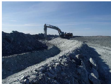
NCIS-116 (2018-07-25), looking SE from Sta. 1+700/+37 m (approx.). Excavation of a 0.8 m (approx.) deep, 1 m wide shallow ditch in the rockfill capping with an excavator from Sta. 1+500 m to 1+455 m.
