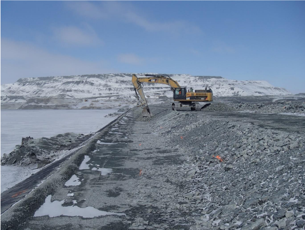
Photograph CD-1838: From Sta 0+835/-20 m, looking N. Placement of a second 0.5 m thick lift of coarse filter from El. 143.5 m to 144 m with an excavator from Sta. 0+500 m to 0+835 m and from 0+930 to 40+730 m.
