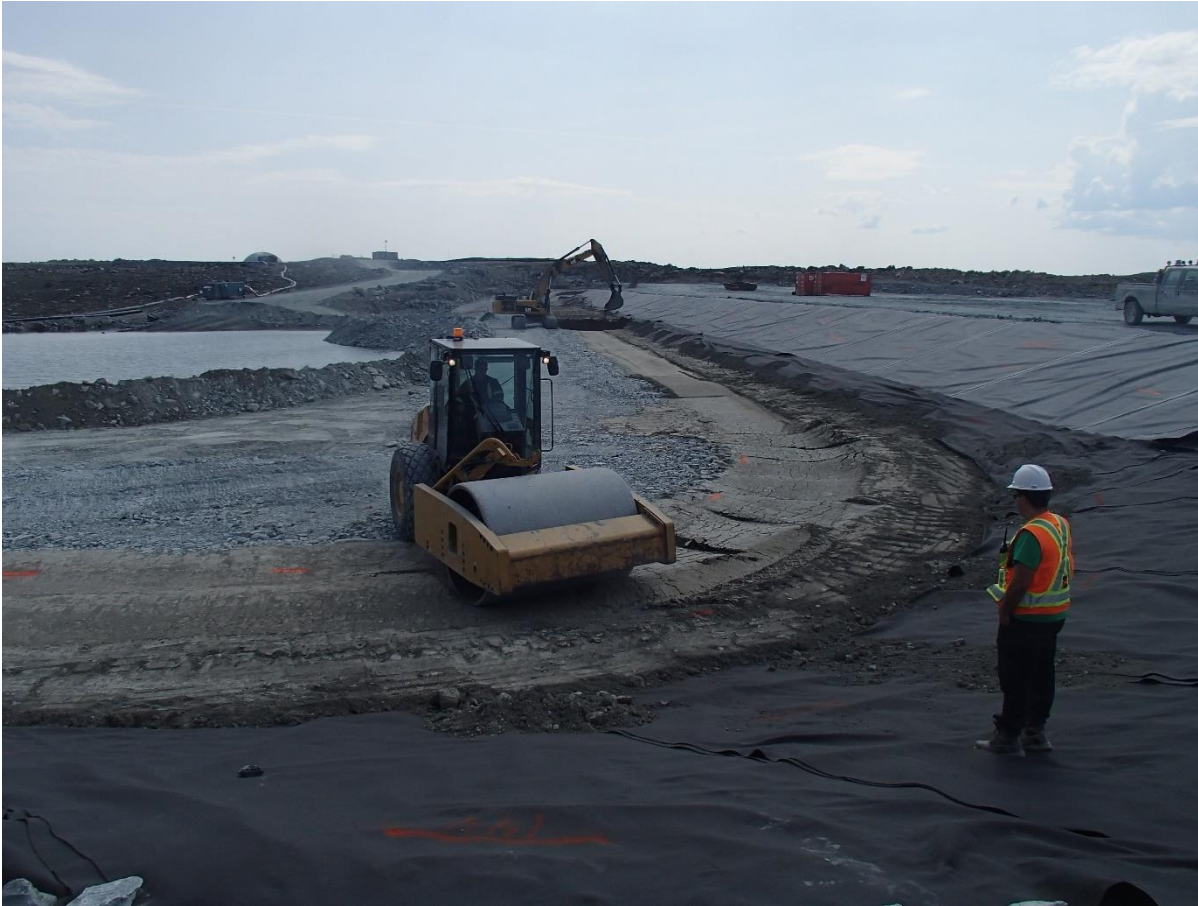
Photograph SD3-328: From Sta. 20+610/-43 m, looking S. Compaction perpendicularly to the longitudinal axe of Saddle Dam 3 of the 0.5 m lift of low quality till (0-150 mm) at El. 142.5 m with a 10-tonne smooth-drum compactor without vibration (4 passes) from Sta. 20+615m to 20+635 m.
