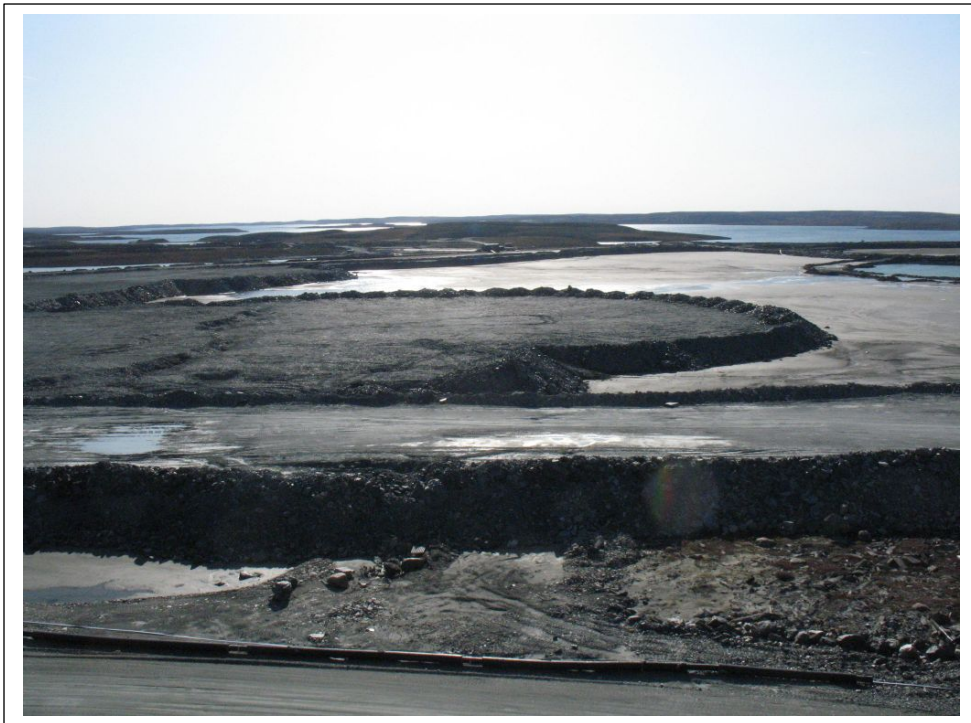
Photo No. 6 Advance of rockfill cover over North Cell of the TSF
