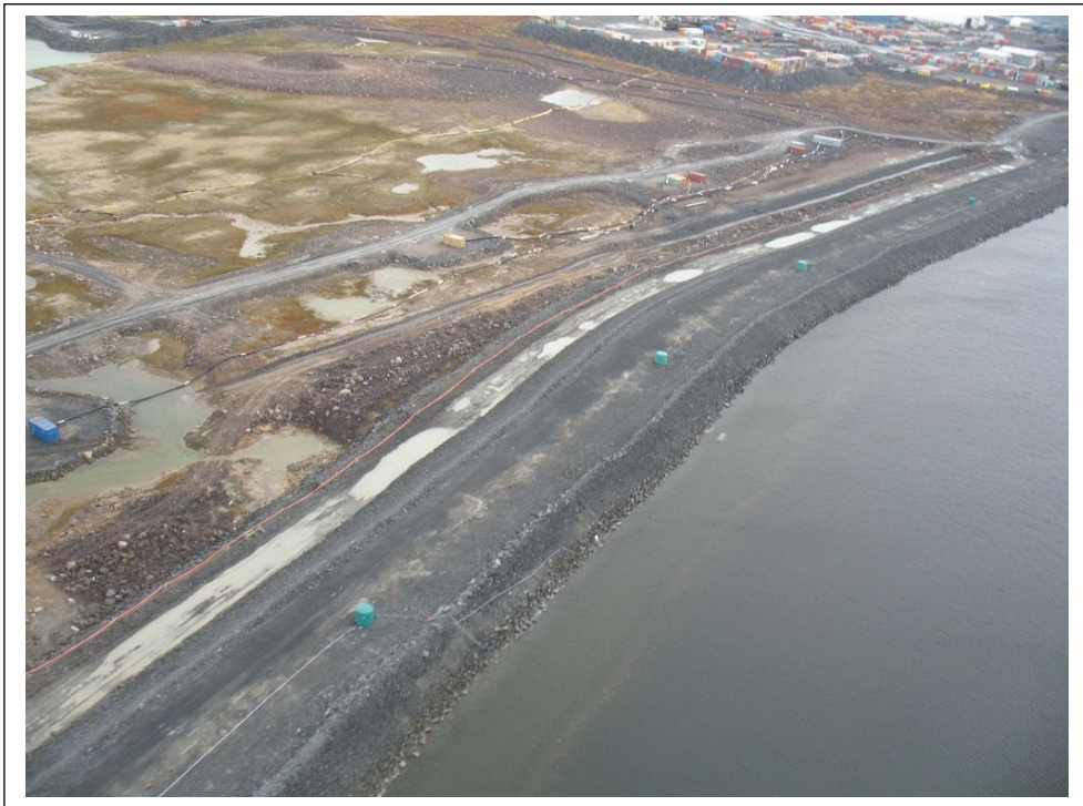
Photo #16 Whale Tail Dike. Seepage collection ditch
