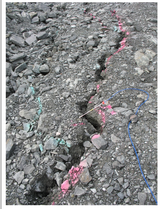
Photo #21 East abutment. Cracking on crest
