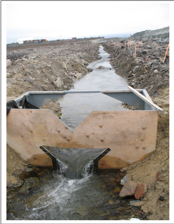
Photo No. 9 V-Notch weir for clean water flow at Stn. 0+430
