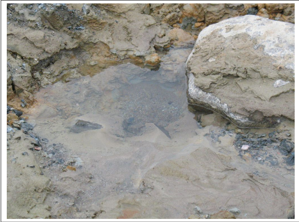
Photo No. 11 Sand boils in western sector
