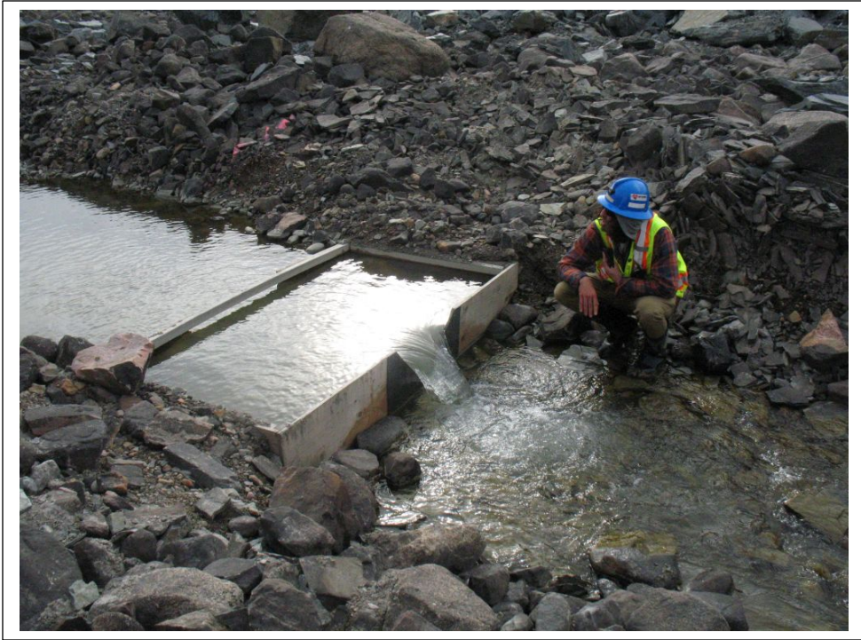
Photo No. 7 V-Notch weir for clean water flow at Stn. 0+560
