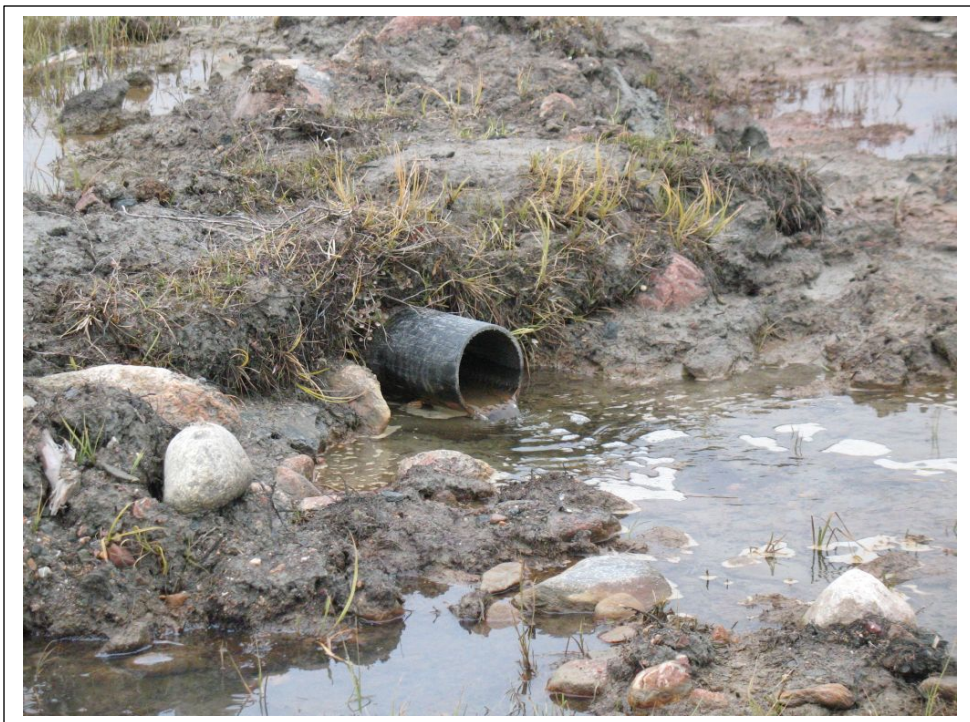
Photo No. 18 Seepage flow from NE Dike
