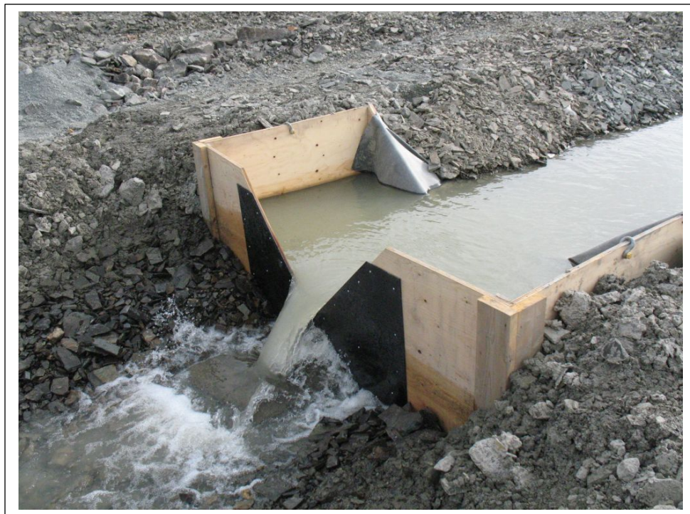
Photo No. 6 V-Notch weir for turbid flow
