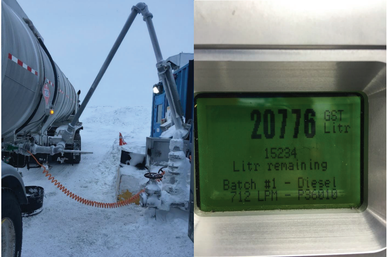
Photo 3: Agnico Eagle Ltd.'s Refueling Station – Loading arm and Scully System
