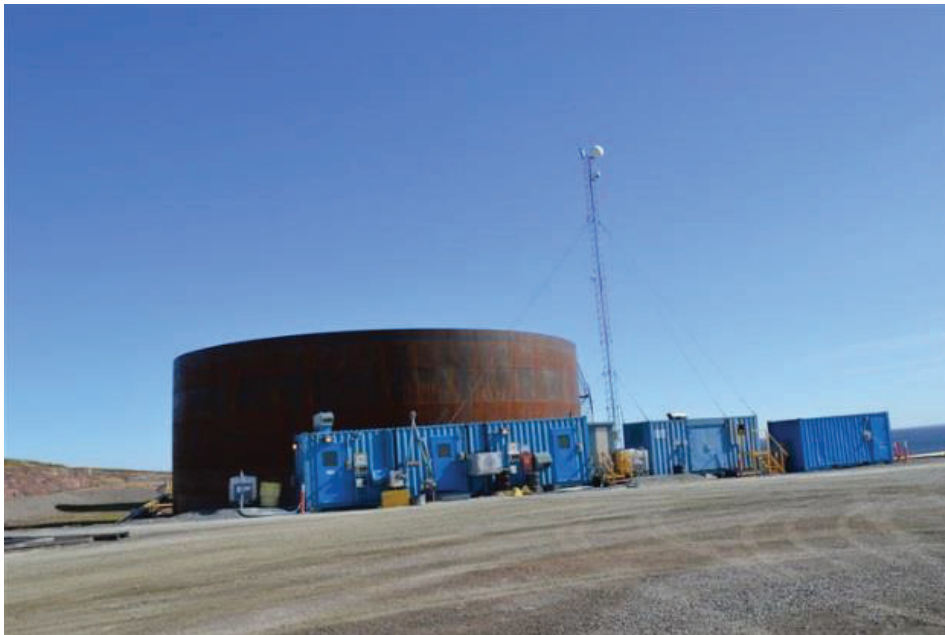
Photo 4: Agnico Eagle Ltd.'s Refueling Station – general view
