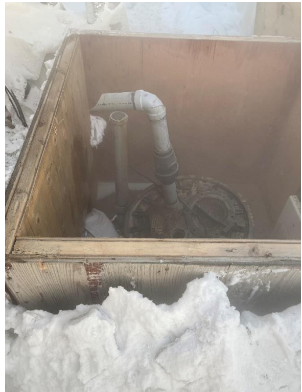
Figure 2. Broken piping causing spill – 2022-02-03
