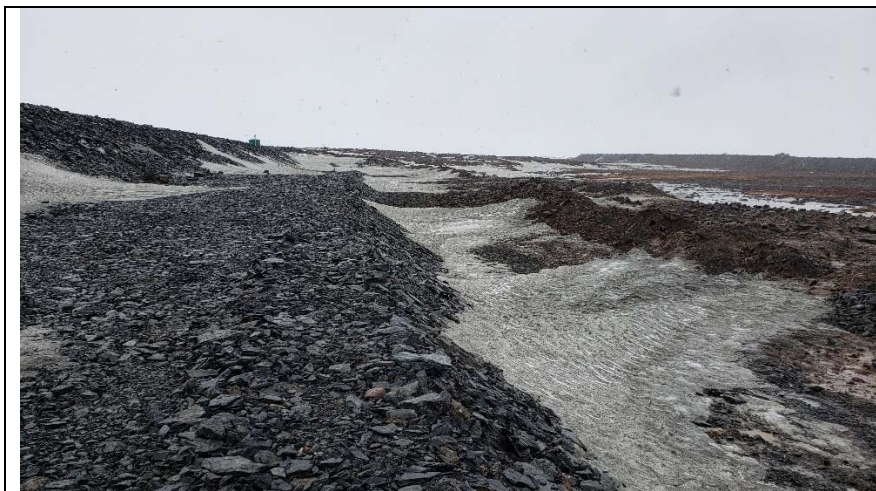
US1: Upstream slope. Water pond far from structure & frozen.
