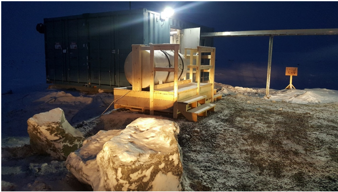
Picture 3 Electrical substation after construction
