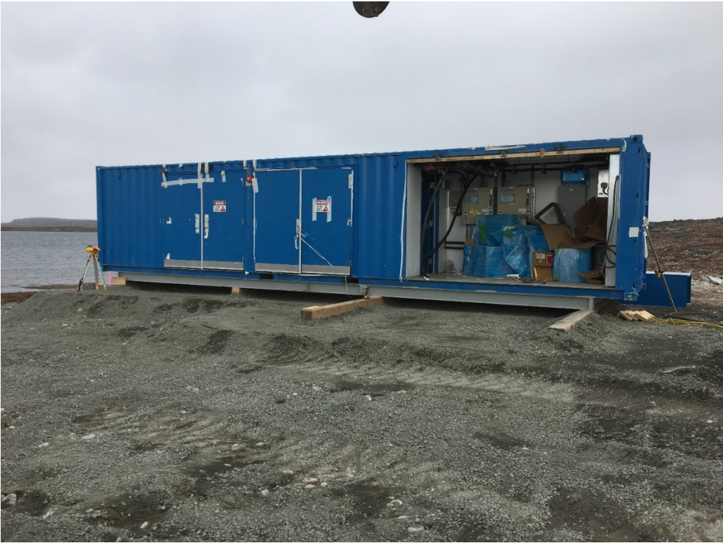
Picture 2 Pump section of pumping station
