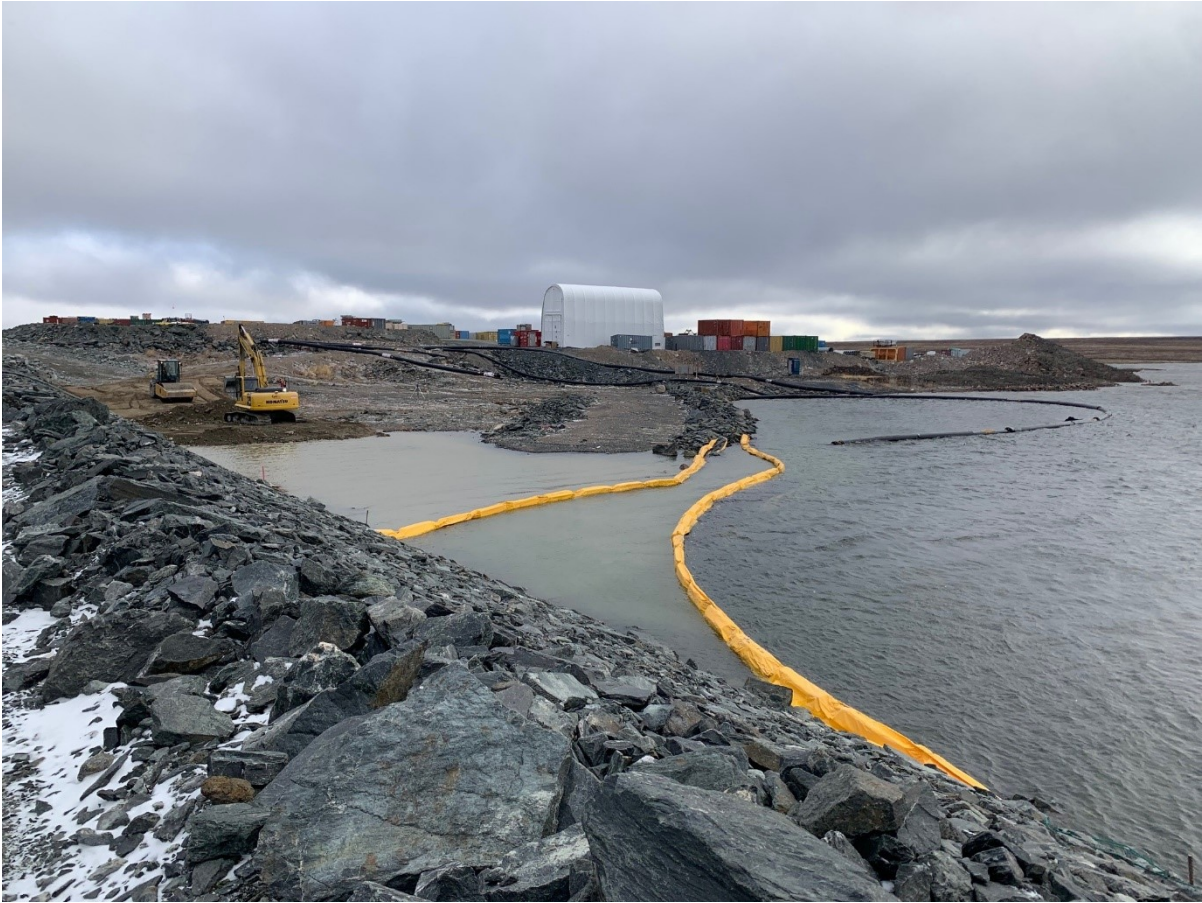
Figure 4. In-water construction for the Whale Tail Dike East Abutment Thermal Berm (September, 2022) showing turbidity curtains.
