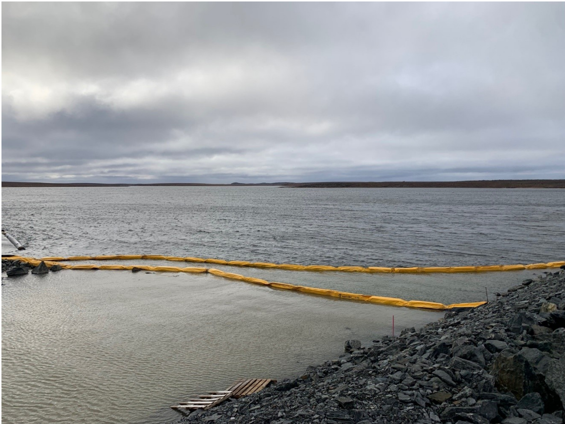
Figure 3. Turbidity curtains deployed during in-water construction for the Whale Tail Dike East Abutment Thermal Berm (September, 2022).
