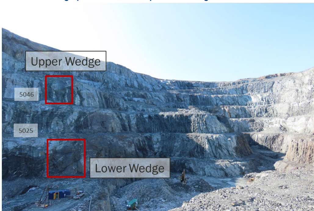
Photograph 6-24: Pit E sump area showing potential wedge instability
