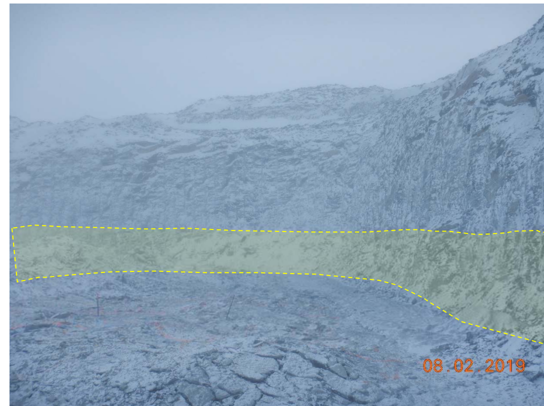
Zone BB14: BB Phaser, South West Wall: Lightly scale the wall and pick up debris.
