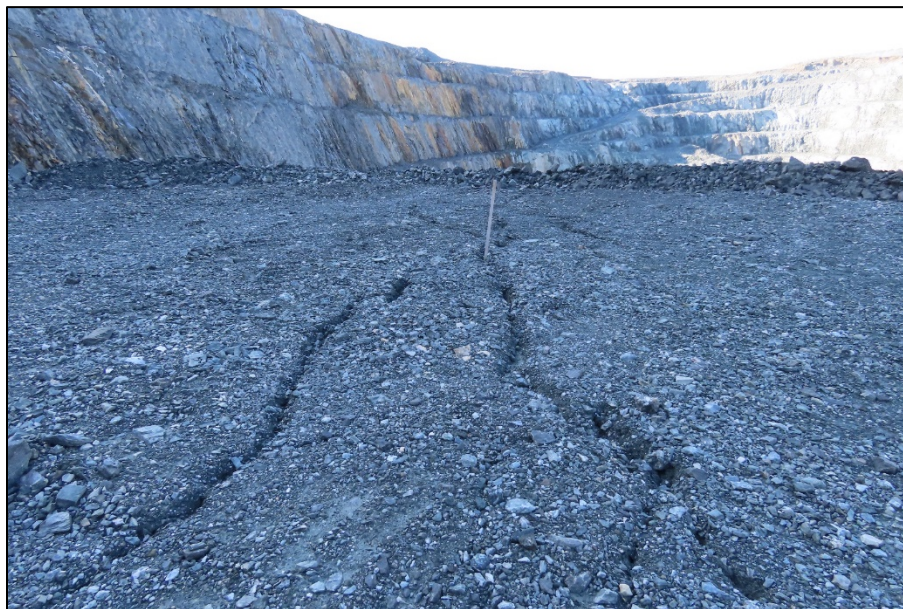
Photograph 5-4: Pit D Dump 5088 mRL platform showing inactive tension cracks
