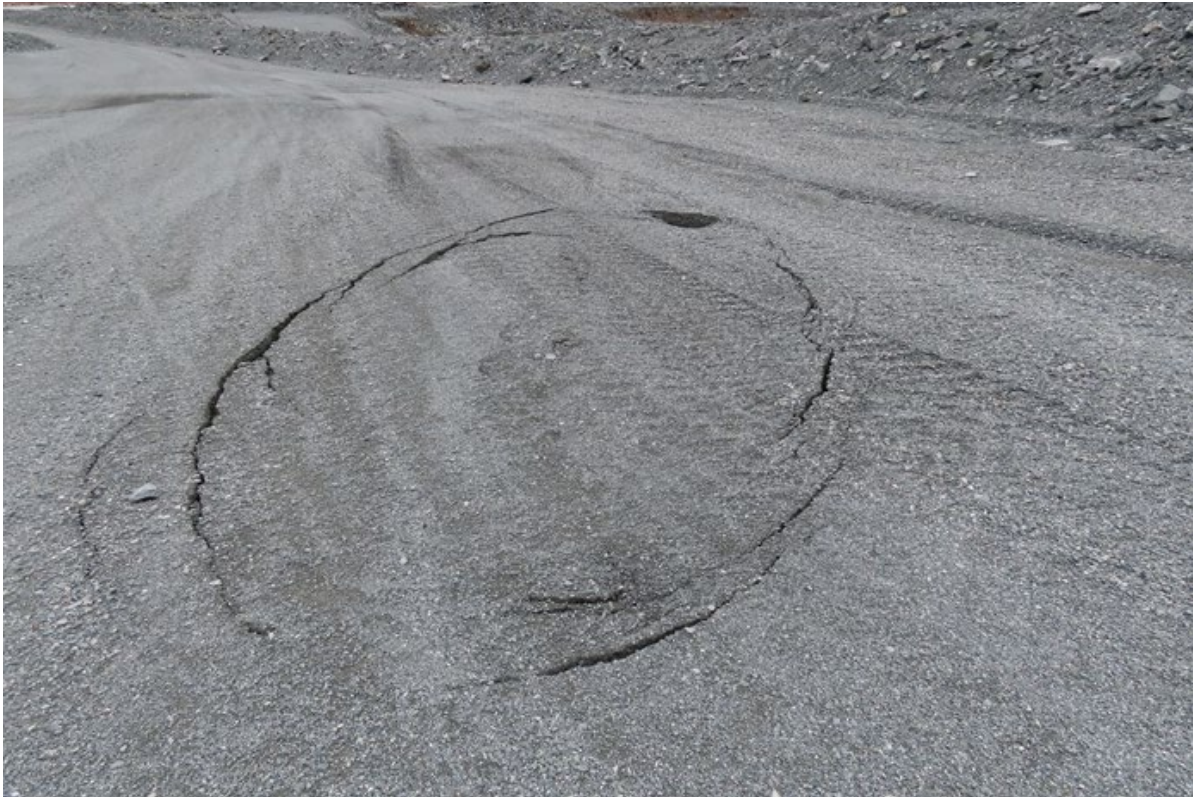
Photograph 8-23: Sinkhole formation on road between BB Phaser and Phaser pits
