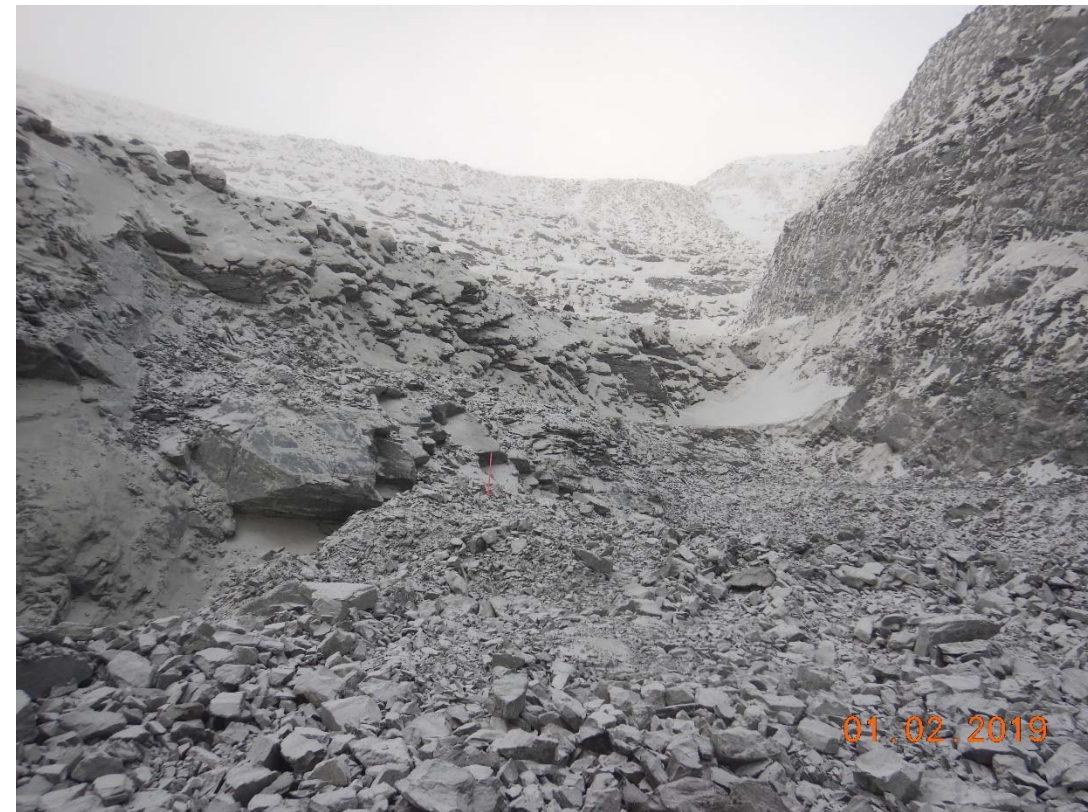
Zone V45: Vault Bottom: No remedial actions required while finishing mucking. Limit on-foot personal access within 10 m of the wall. (West wall)
