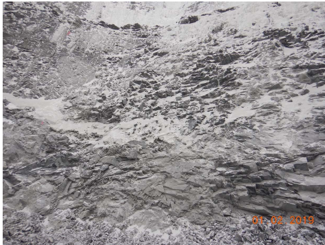
Zone V45: Vault Bottom: No remedial actions required while finishing mucking. Limit on-foot personal access within 10 m of the wall. (East Wall)
