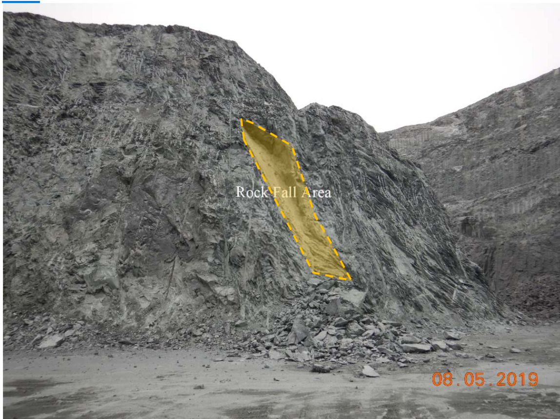
Fig.1: Photo taken after rock fall was reported.
