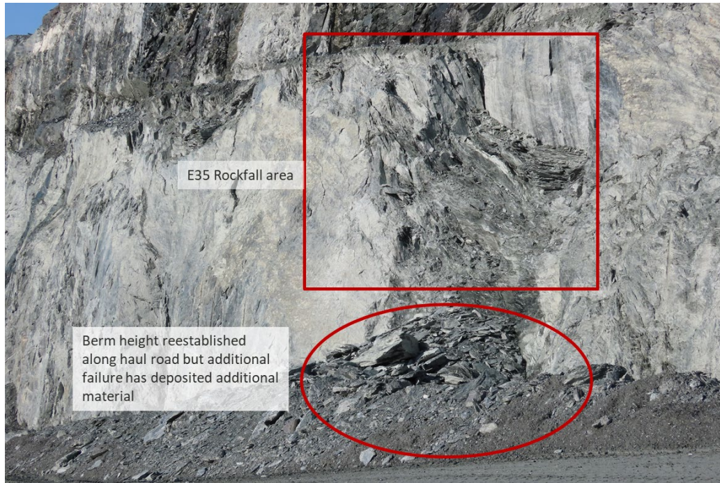
Photograph 6-17: Zone E35 rockfall
