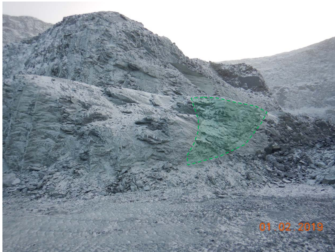
Zone E54: E5, East Wall: Potential wedge was investigated with the shovel and stayed in place.
