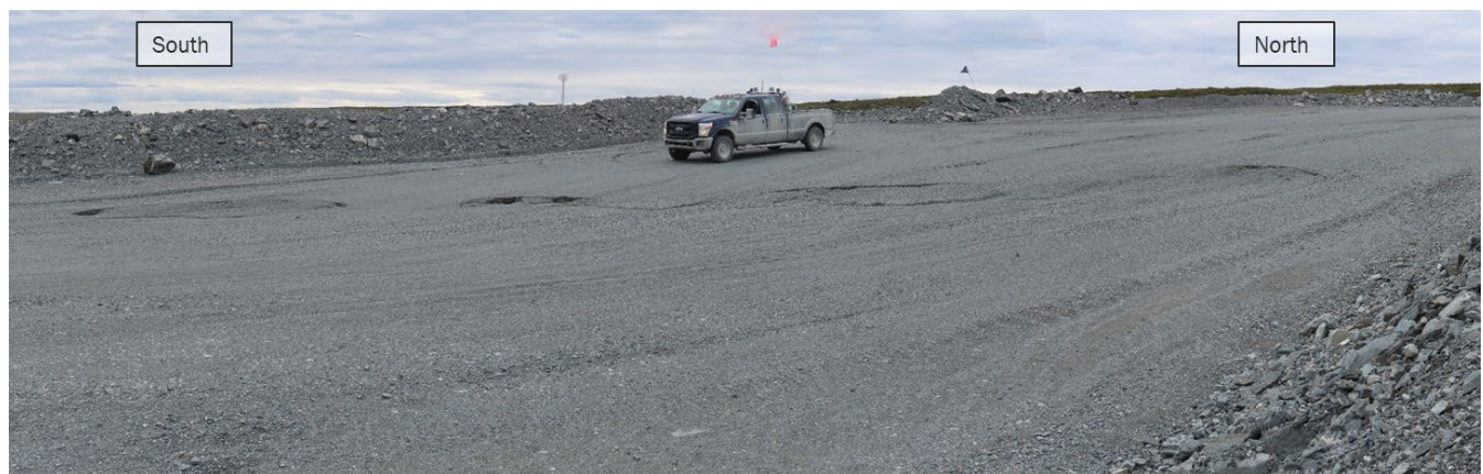
Photograph 8-22: Sinkhole development and settlement of road surface between Phaser Pit and BB Phaser Pit
