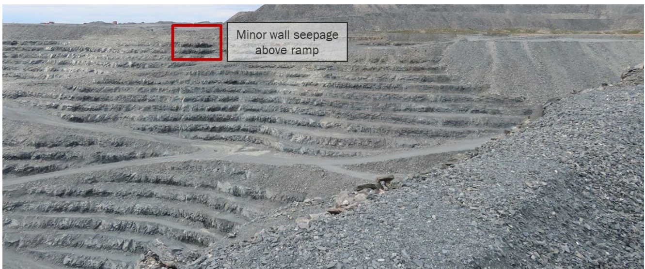
Photograph 8-1: Minor wall seepage noted on west footwall of Vault Pit (2019)
