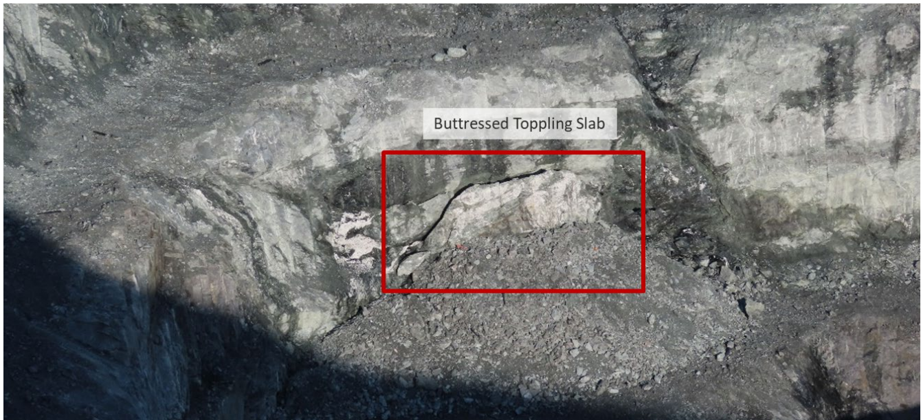
Photograph 6-5: Buttressed toppling slab in the south wall of Pit E
