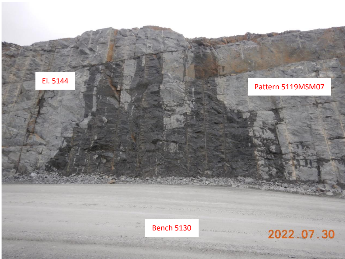
Photo 1: Pit seepage along Whale Tail Pit south wall, concentrated water source type, flowing joint (water source is related to ongoing water management operations), looking south (July 30, 2022).
