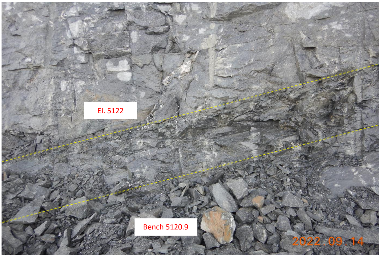
Photo 6: Whale Tail Pit P3, looking southwest; water flowing from a fault or brittle structure (September 14, 2022).
