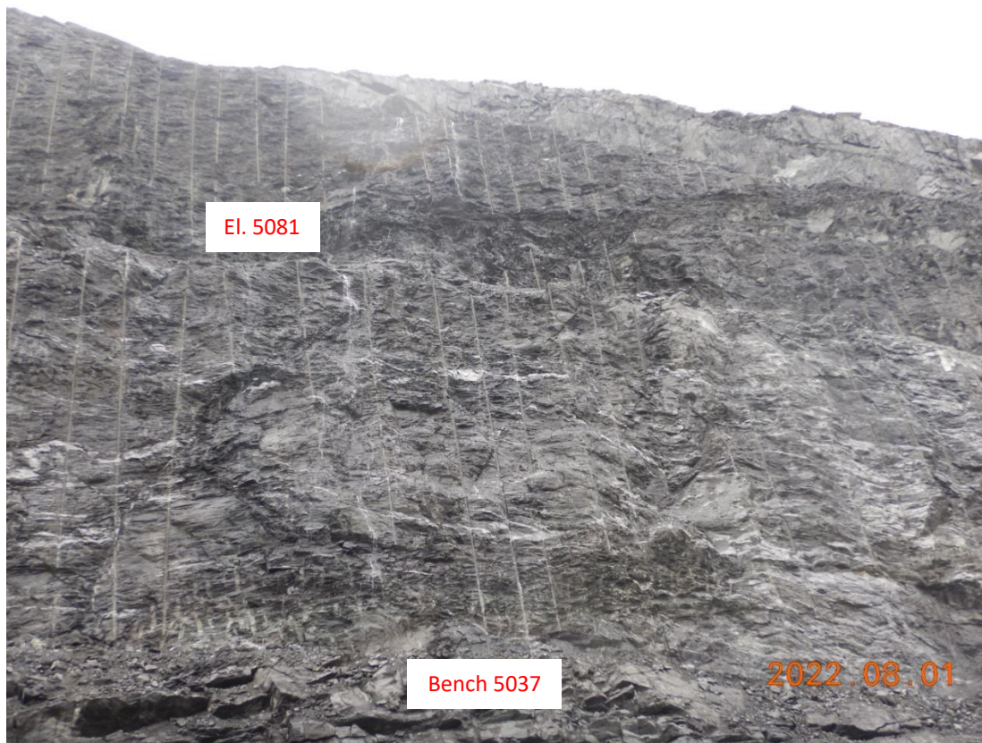
Photo 3: Pit seepage along Whale Tail Pit south wall; flow coming from the ramp during a rainy day but precipitation does not justify the amount of concentrated water (August 1, 2022).
