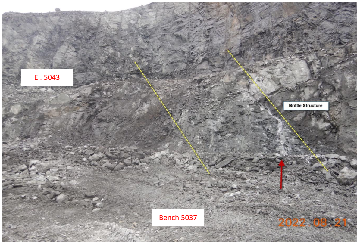
Photo 5: Whale Tail Pit P1, looking southeast; water was flowing steady from the eastern end of WHL P1, and this condition was ongoing for a couple weeks prior to August 21, 2022; water was observed flowing through a brittle structure (see red arrow), and the source is likely the same that forms the ice wall during sub-zero conditions, and flows underneath the ramp and exits through the wall (August 21, 2022).
