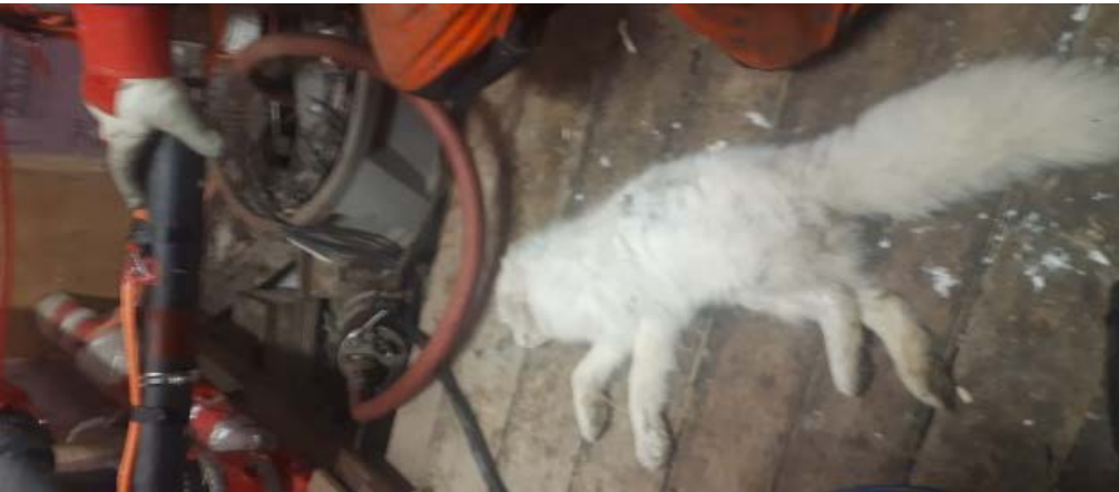
Artic fox removed from the grease trap
