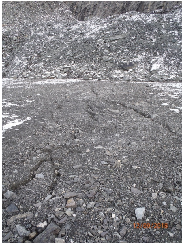
Photograph 5-4: D Dump radial tension cracks
