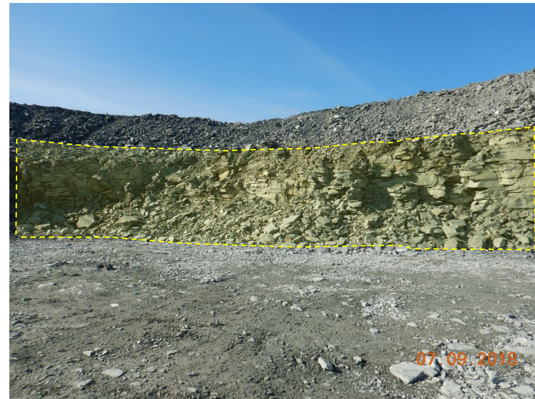
Zone BB04: E4, West Wall: Lightly scale the wall, and pick up debris.
