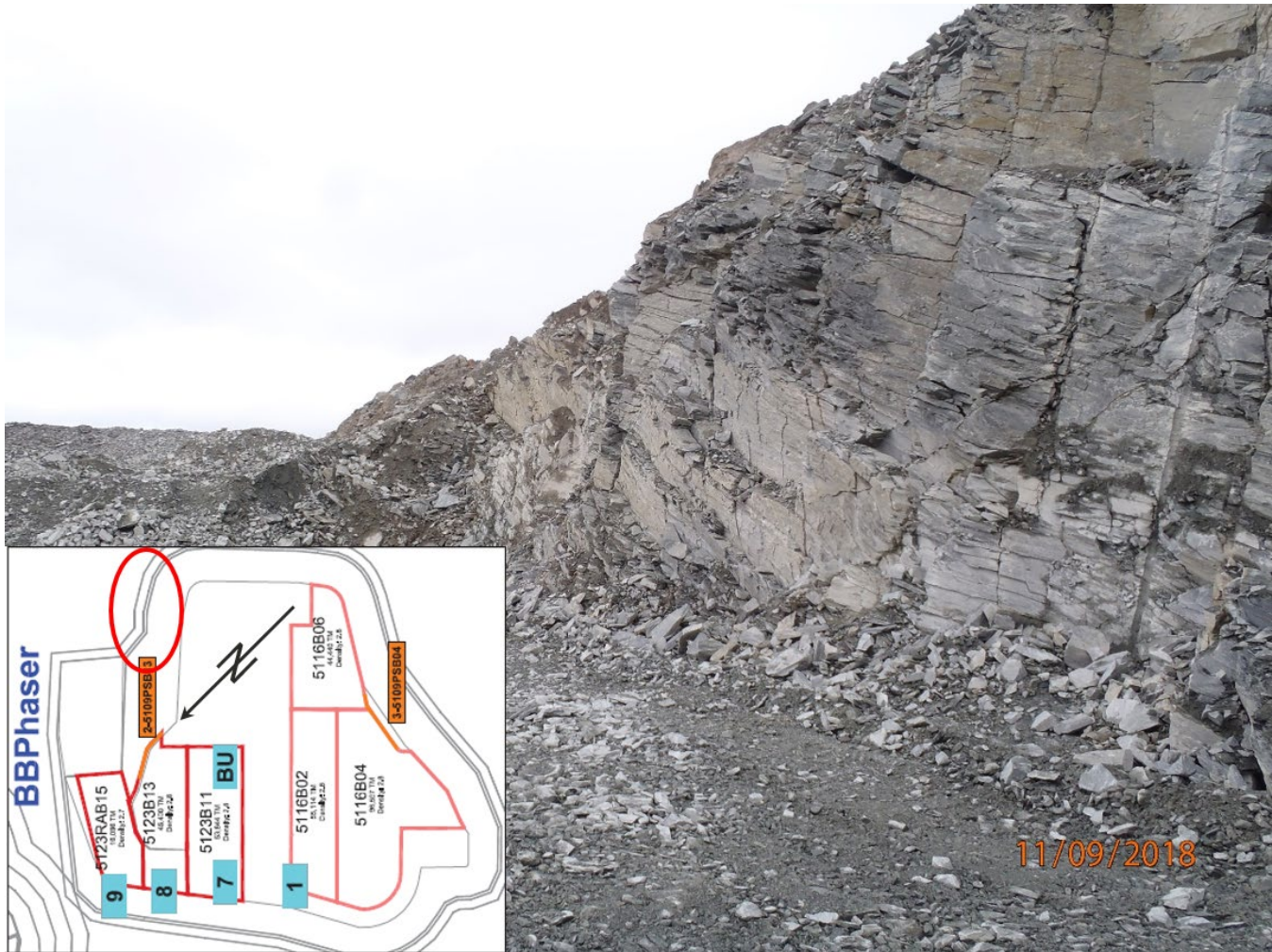
Photograph 8-21: BB Phaser Pit east to north end wall showing continuous orthogonal joint surfaces
