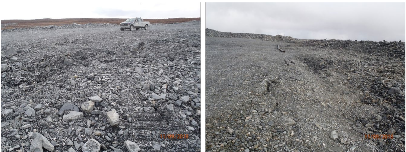
Photograph 8-18: Thermal cap showing hummocky ground, differential settlement, and voids
