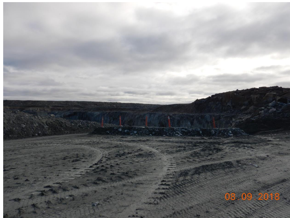
Zone E29: E5, South Wall: Restricted Access while waiting for the rock fall removal.
