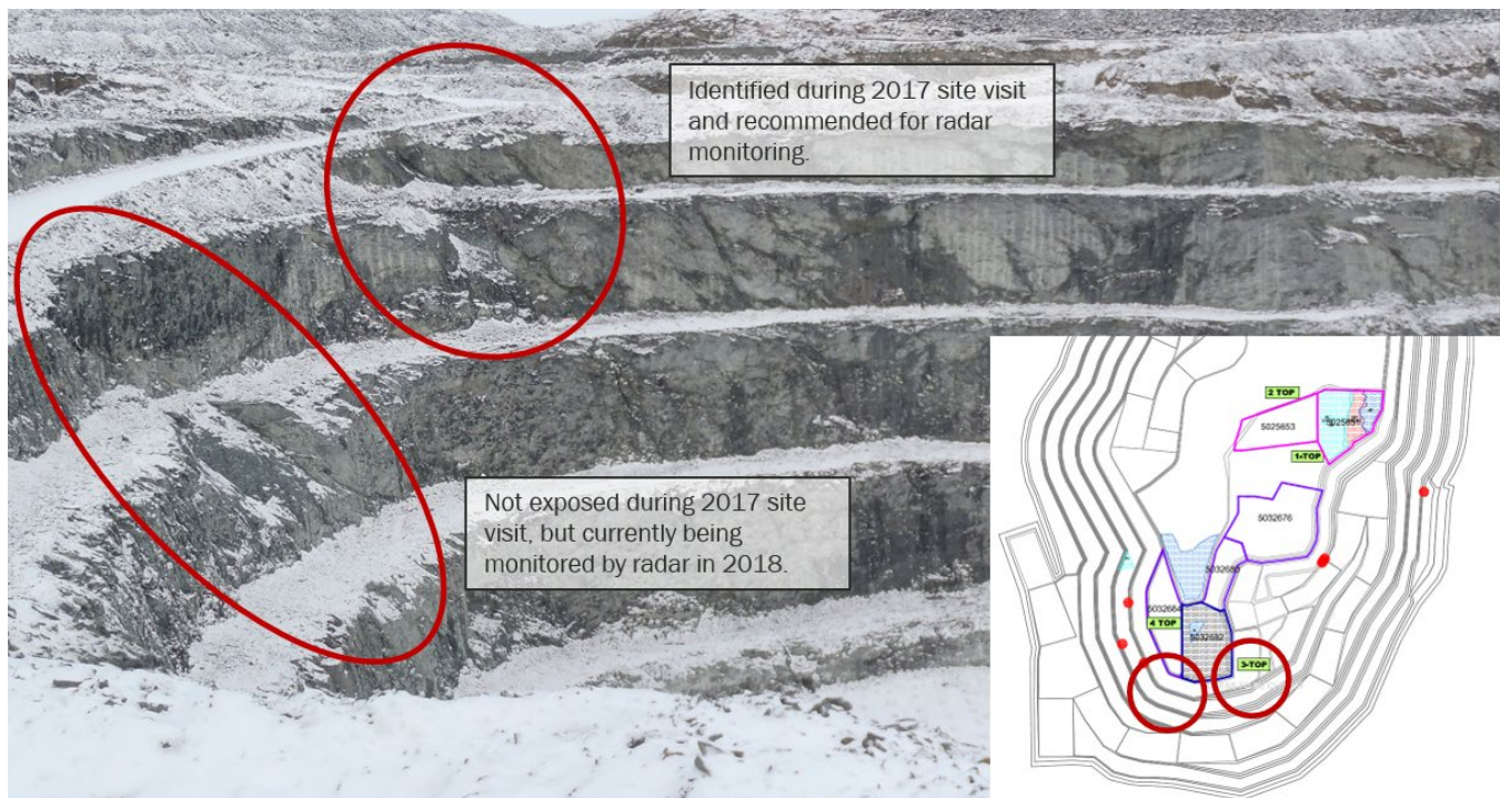
Photograph 6-5: North to northwest dipping shear planes contributing to wedge and planar instability in south wall
