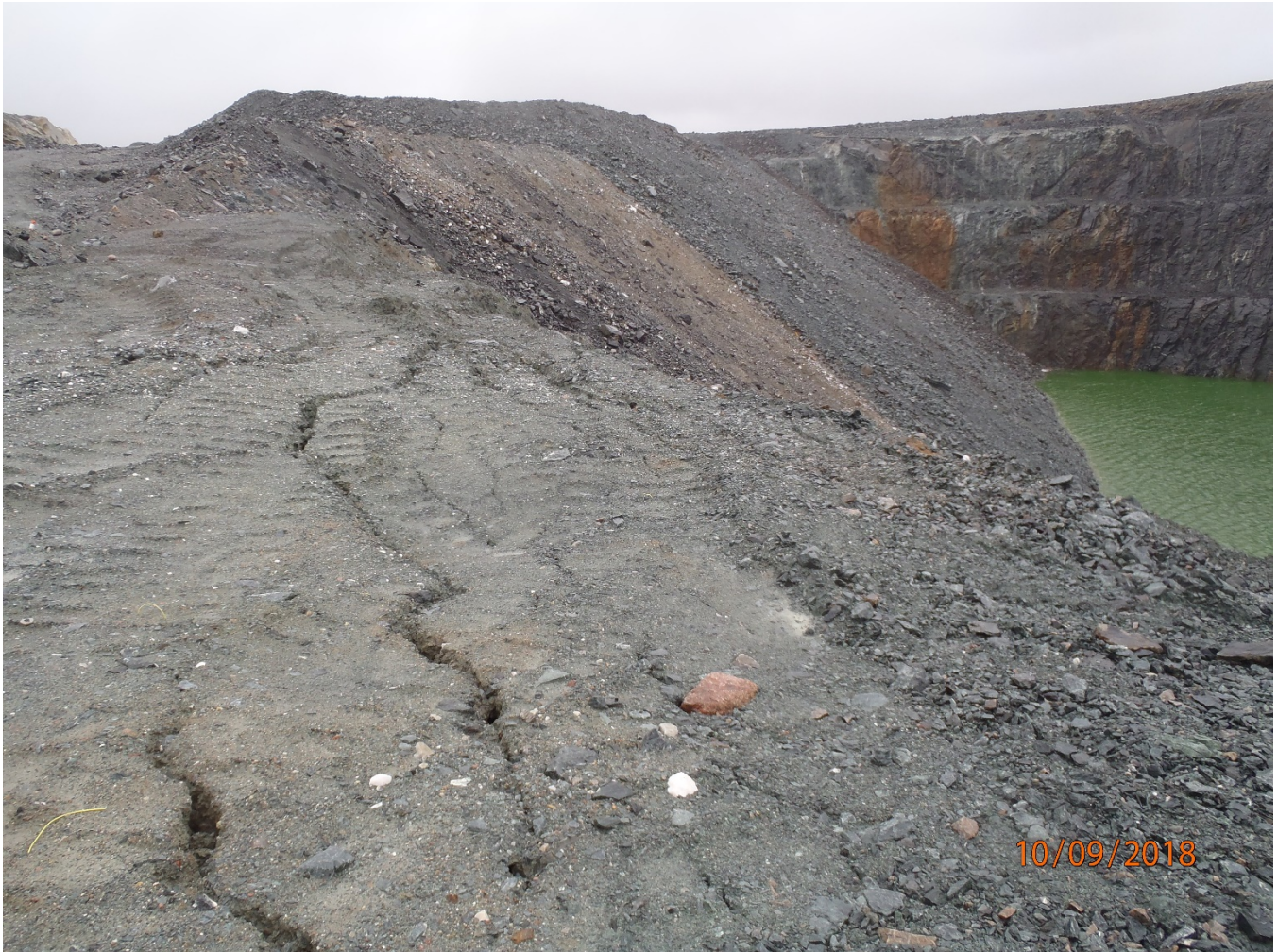
Photograph 7-7: Tension cracks at crest of Goose South Dump
