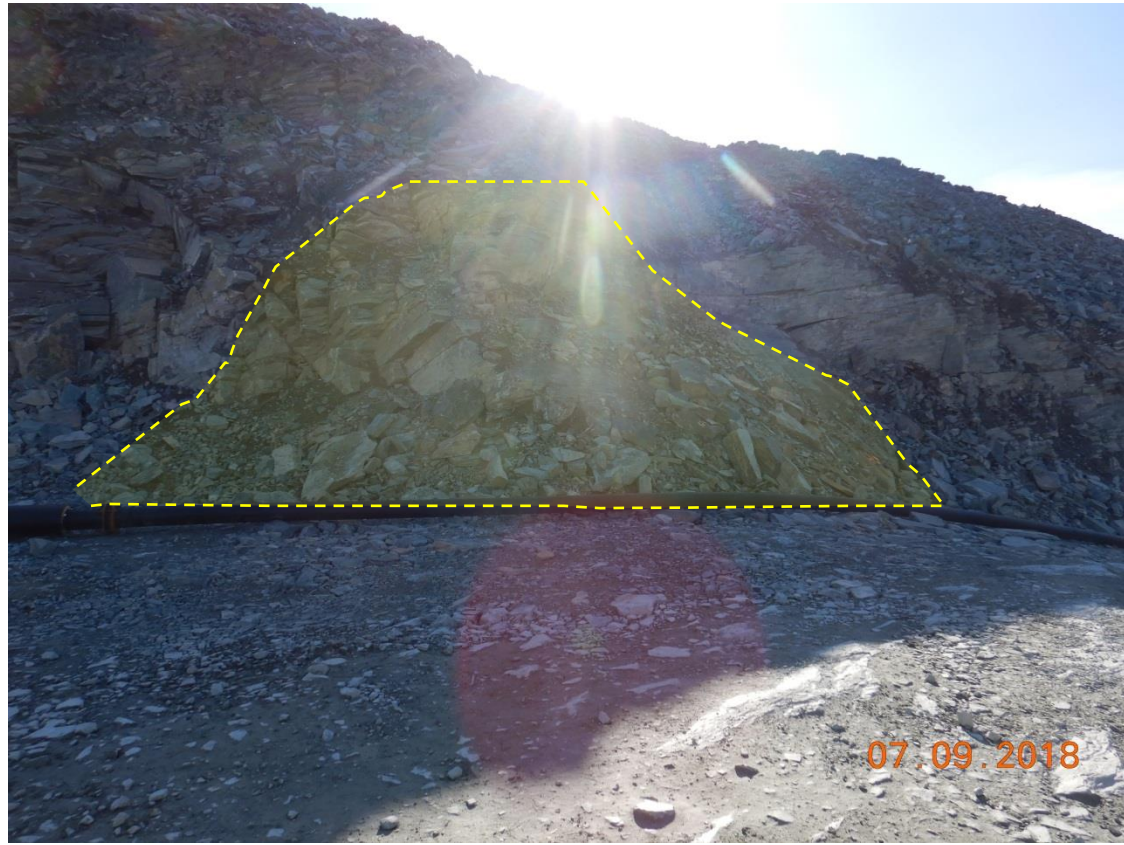
Zone BB04: BB Phaser East Wall: scale the loose material and remove the bulging section.
