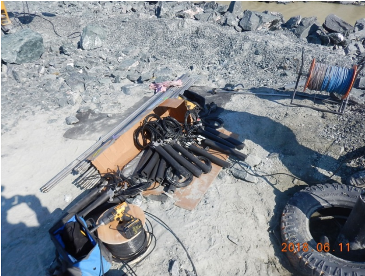
Photo 3.4 : Sensors, cables and Connecting Tube before being assembled
