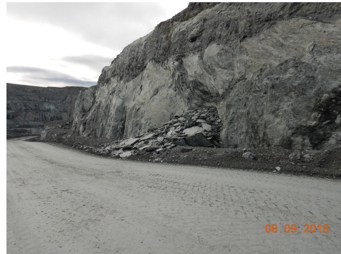
Zone E35: E3 Ramp, West Wall: Remove all loose material from previous rock fall.
