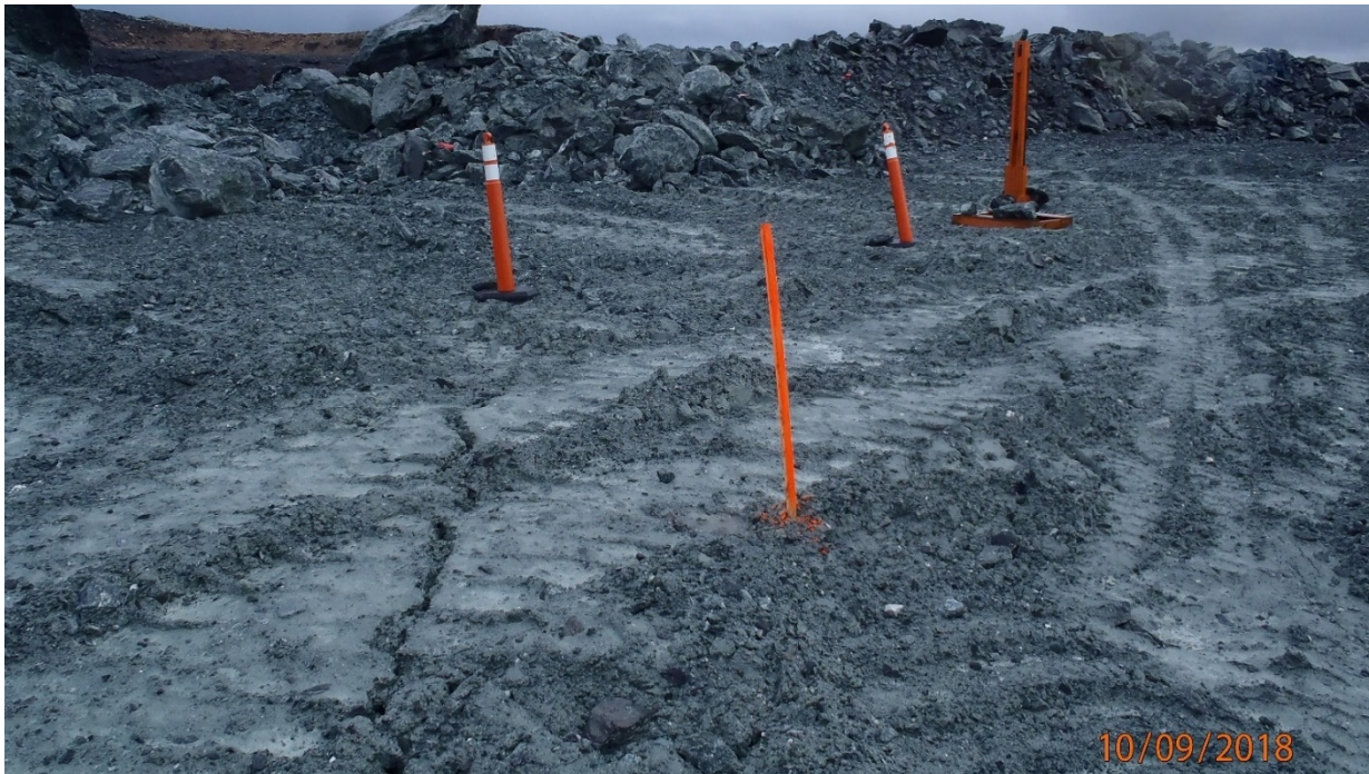
Photograph 4-14: B Dump platform showing sag, tension cracks, and simple wireline extensometer
