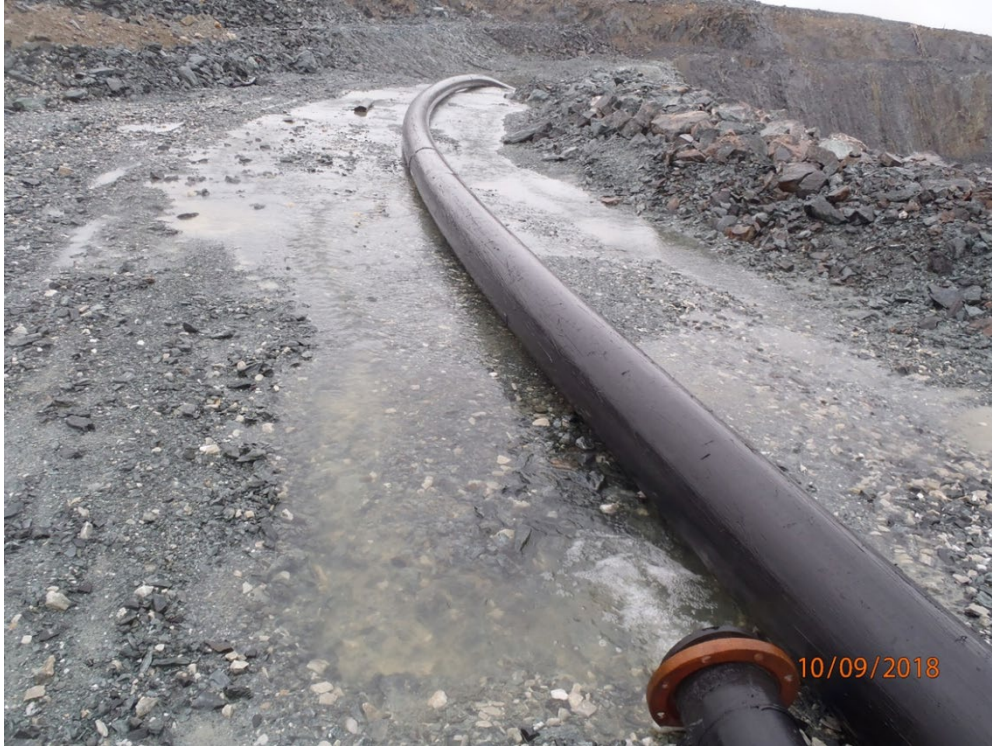
Photograph 7-10: Goose Pit uncontrolled water discharge along north crest
