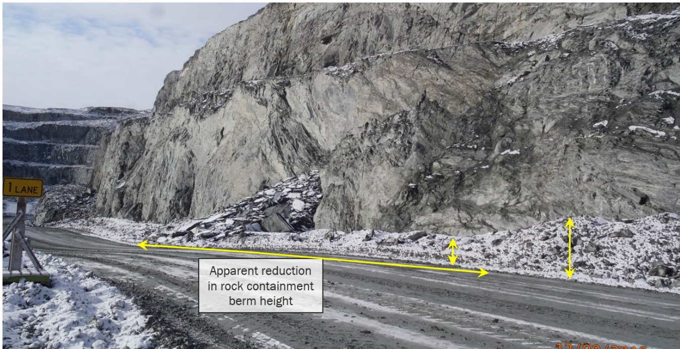
Photograph 6-19: Zone E35 rock fall
