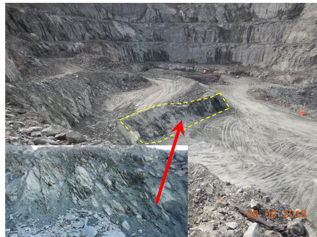
Zone E37: E5, South Wall: Scale and slope the wall. Pull back the bumpers away from the crest.
