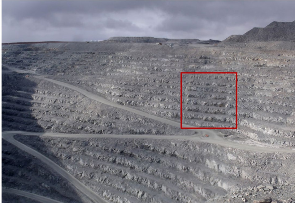
Photograph 8-3: Vault Pit west wall seepage (dry in 2018)
