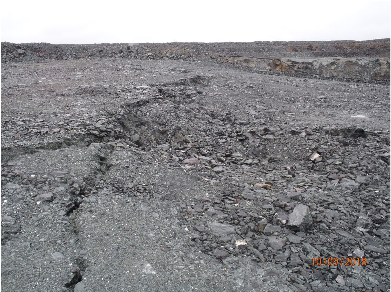
Photograph 7-8: Tension cracks at crest of Goose North Dump
