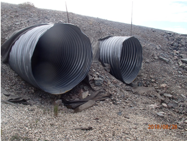
Photograph D1-2: PC-17A km 8+830
