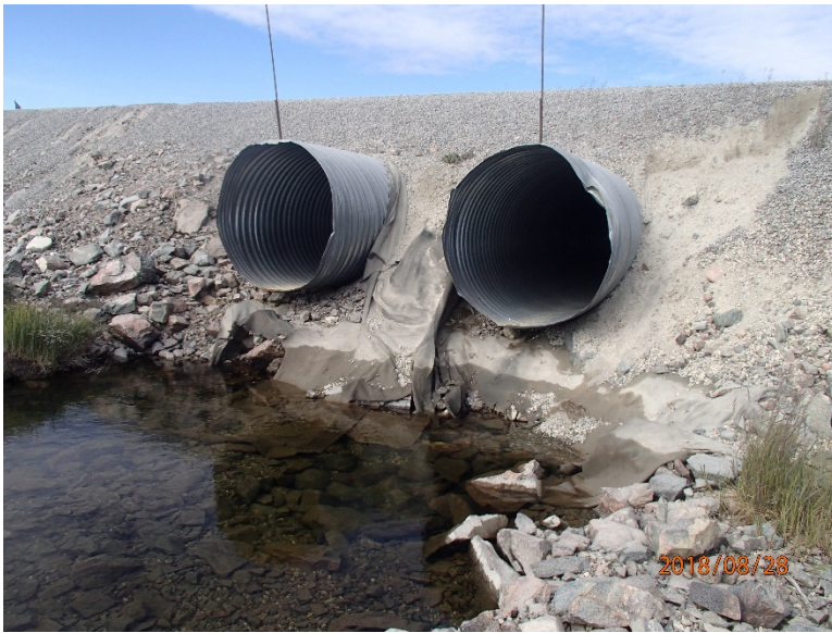
Photograph D1-3: PC-17A km 8+830
