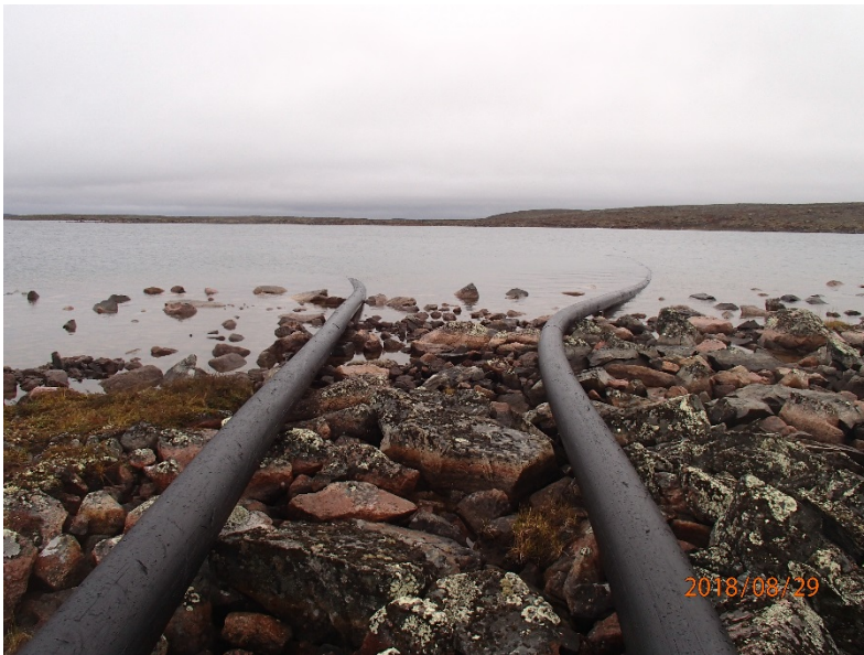
Photograph H4-1 Diffusers – Vault Diffuser
