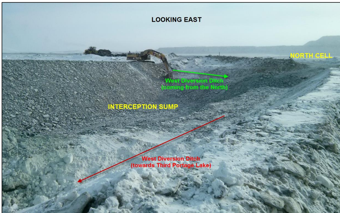
Figure 2-5: North Cell West Diversion ditch interception sump
