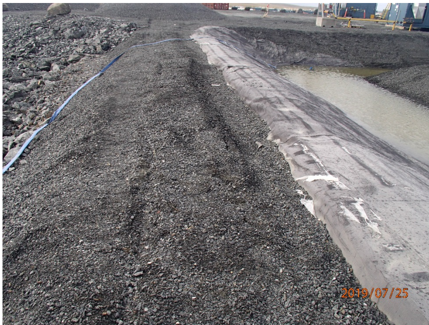
Photograph G3-6 Amaruq Tank Farm
