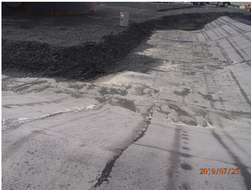
Photograph G3-8 Amaruq Tank Farm
