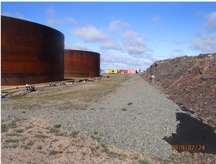
Photograph G1-12 Baker Lake Tank Farm
