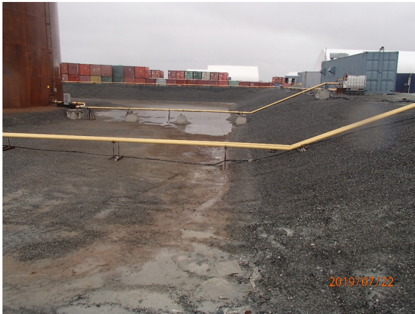
Photograph G2-5 Meadowbank Tank Farm
