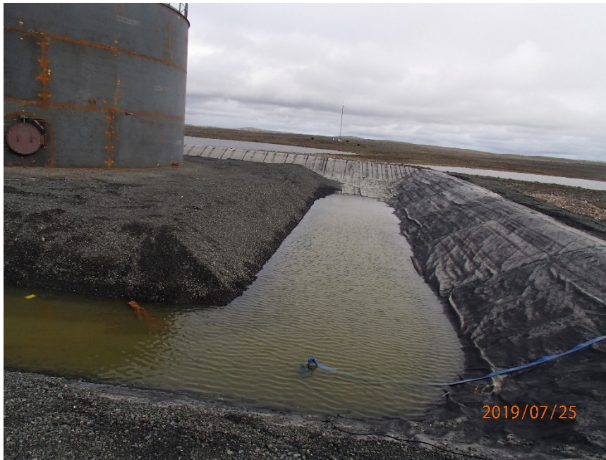
Photograph G3-5 Amaruq Tank Farm
