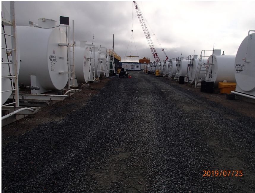
Photograph G3-3 Amaruq Tank Farm
