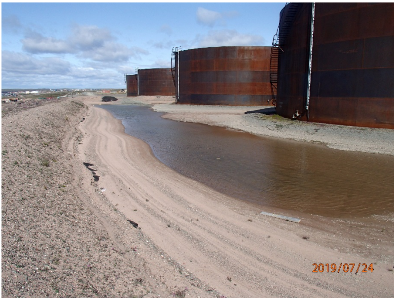
Photograph G1-8 Baker Lake Tank Farm
