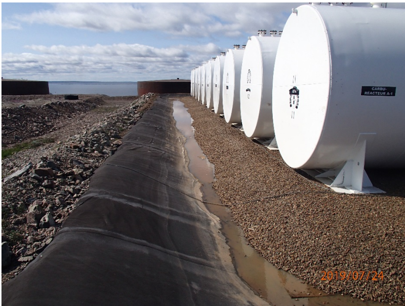
Photograph G1-20 Baker Lake Tank Farm
