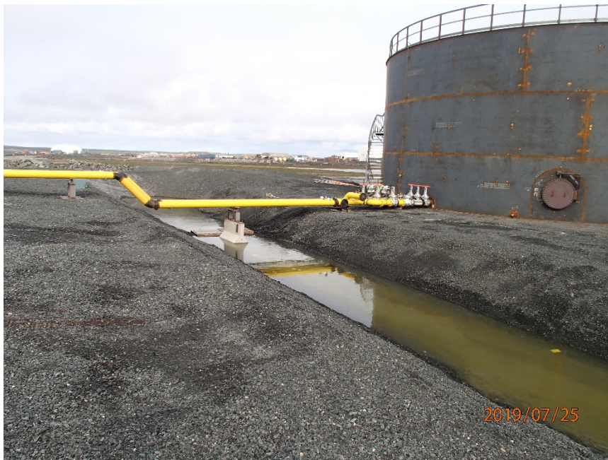
Photograph G3-4 Amaruq Tank Farm
