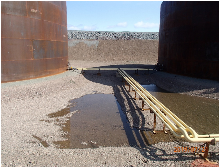
Photograph G1-15 Baker Lake Tank Farm
