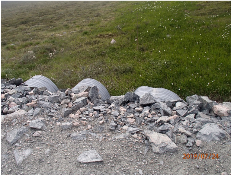
Photograph D2-5: R-18A km 80+950
