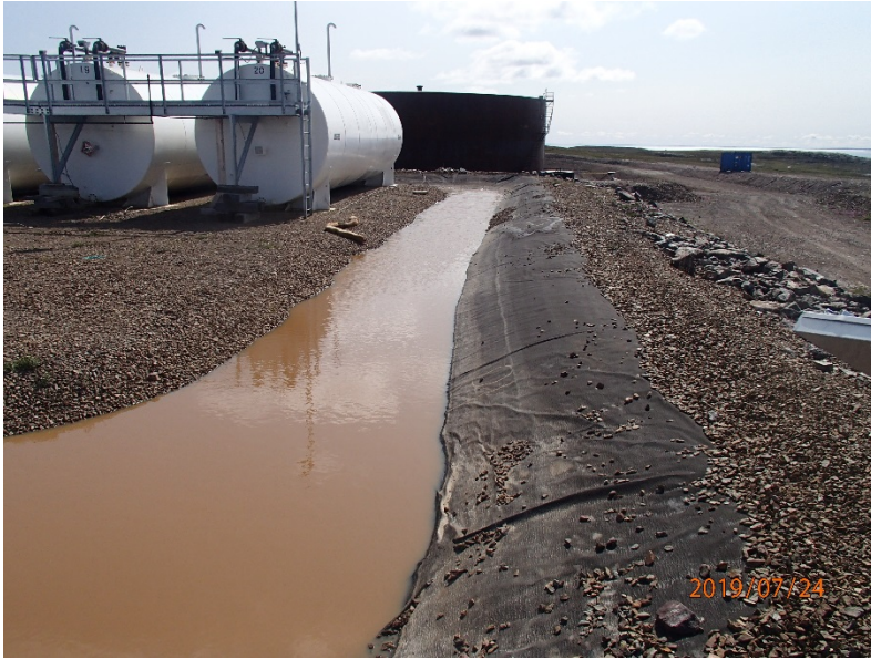
Photograph G1-23 Baker Lake Tank Farm
