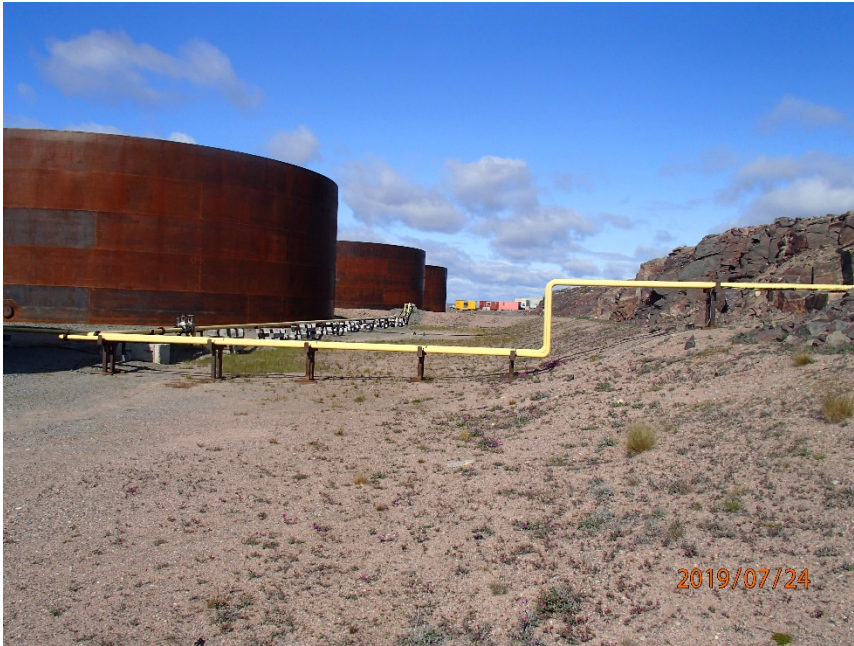
Photograph G1-11 Baker Lake Tank Farm
