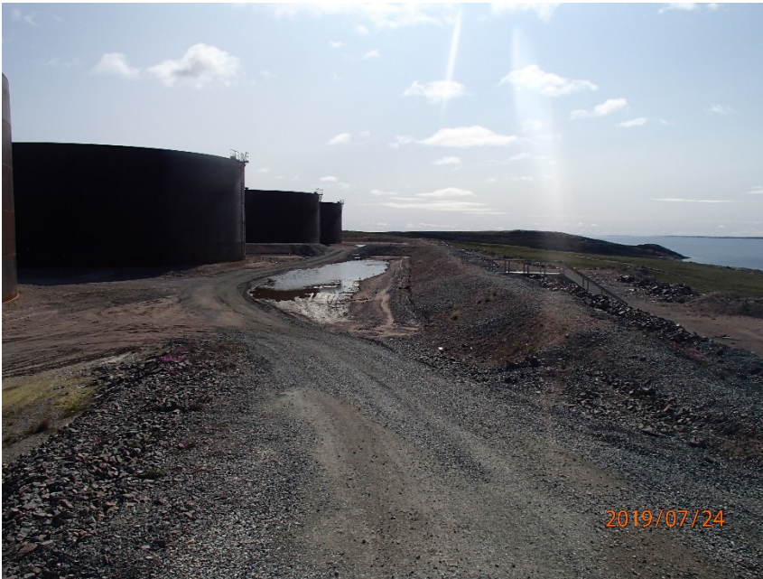
Photograph G1-2 Baker Lake Tank Farm
