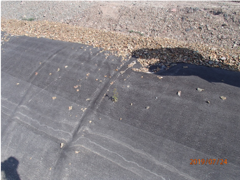
Photograph G1-22 Baker Lake Tank Farm
