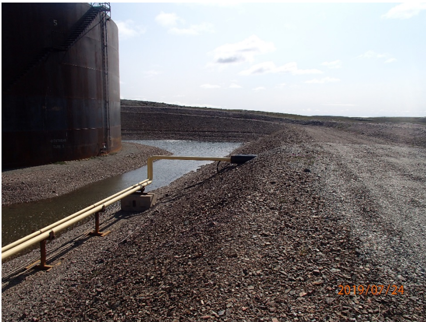
Photograph G1-16 Baker Lake Tank Farm
