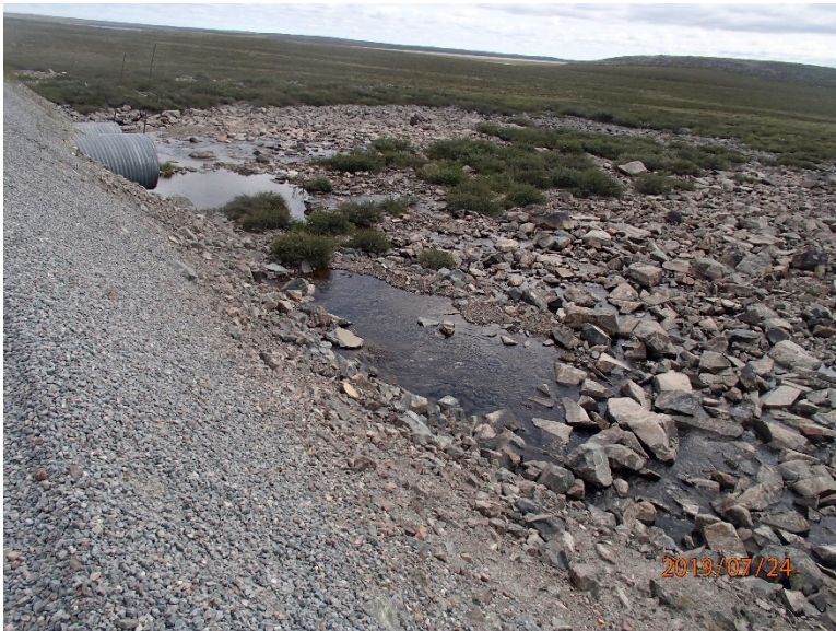
Photograph D2-2: PC-17A km 8+830
