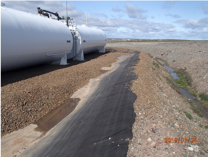
Photograph G1-21 Baker Lake Tank Farm
