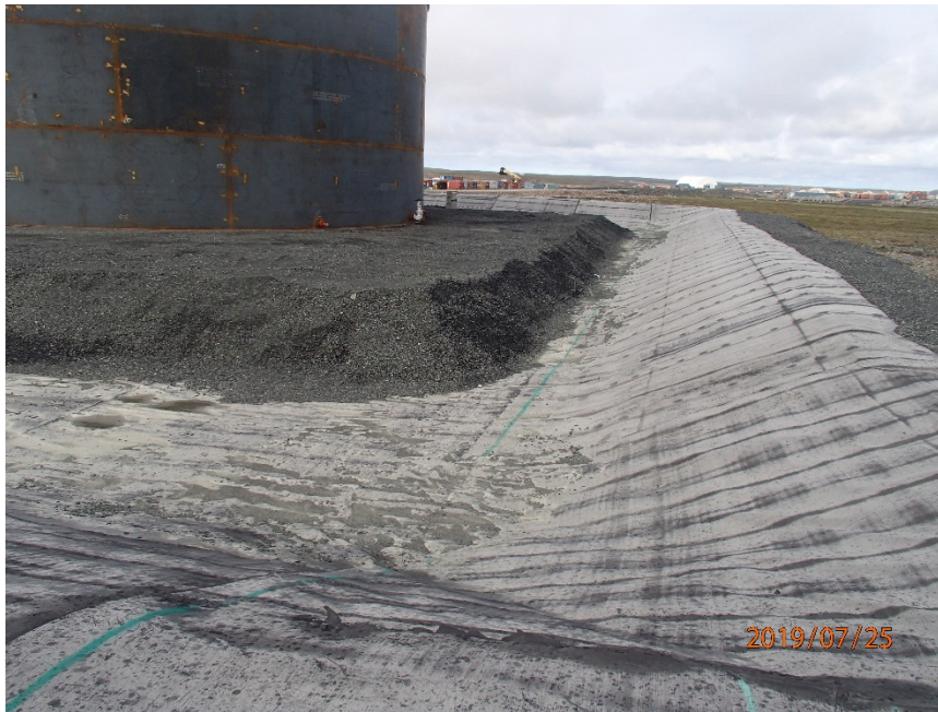
Photograph G3-7 Amaruq Tank Farm
