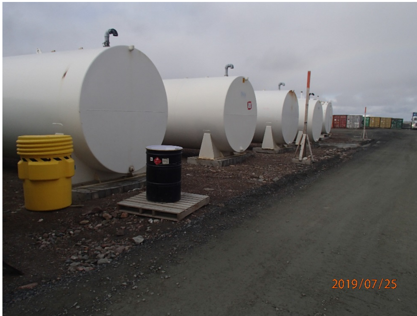
Photograph G3-1 Amaruq Tank Farm
