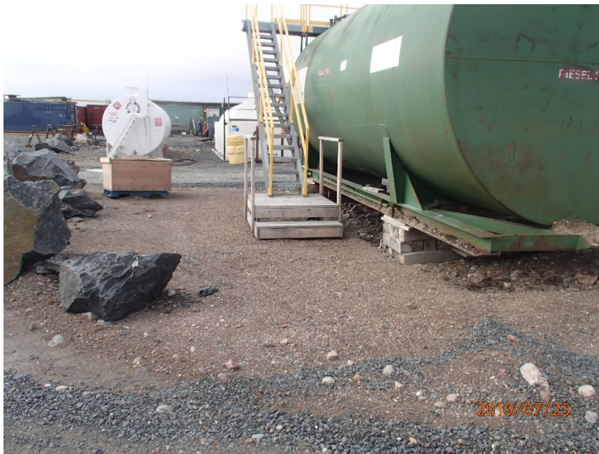
Photograph G3-2 Amaruq Tank Farm
