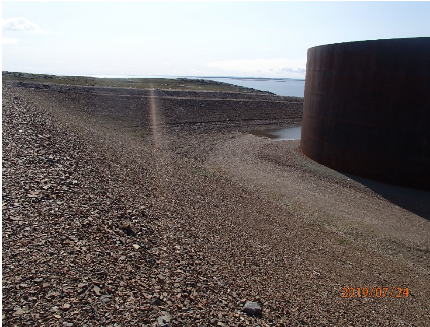
Photograph G1-17 Baker Lake Tank Farm
