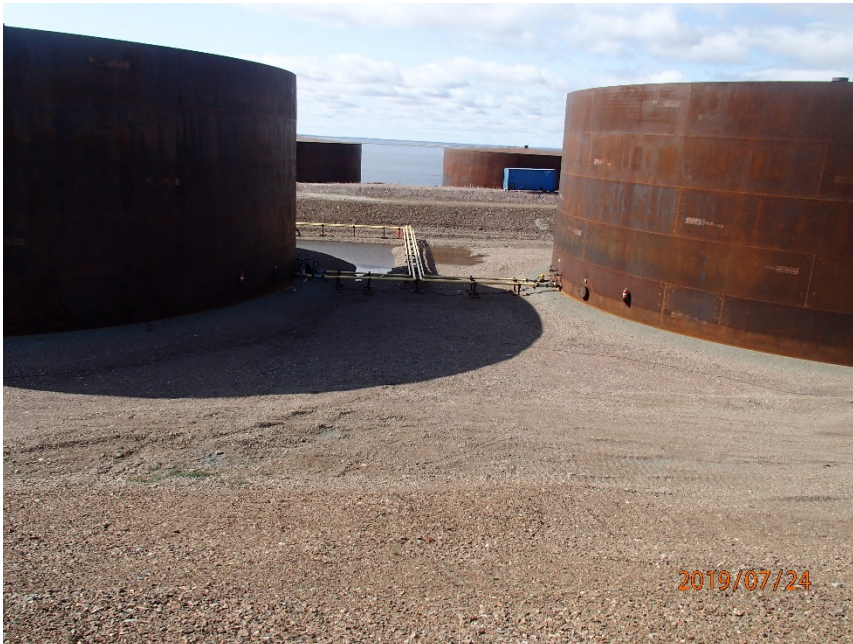
Photograph G1-18 Baker Lake Tank Farm
