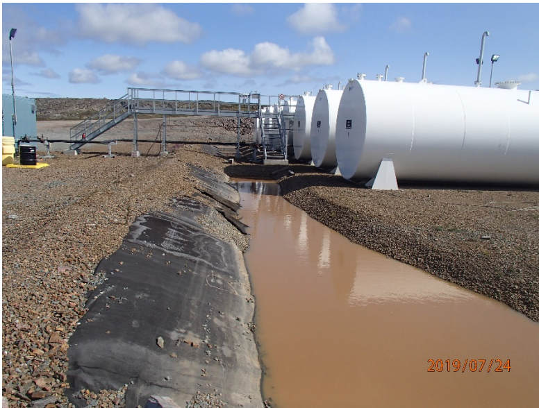
Photograph G1-24 Baker Lake Tank Farm
