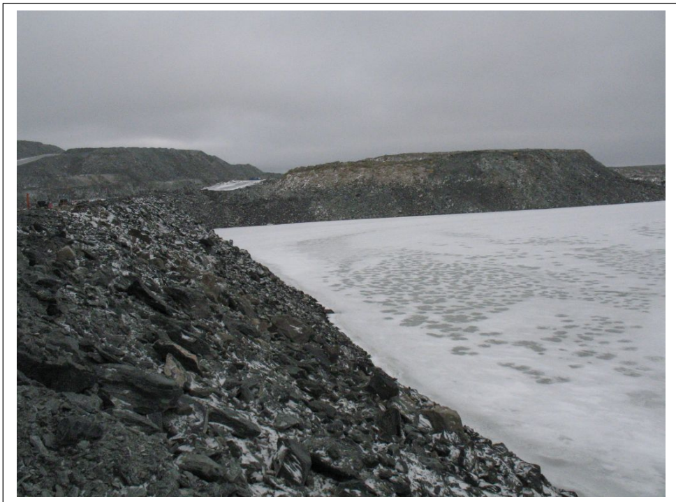
Photo No. 2 South cell supernatant pond at toe of Stormwater dike. View to East.
