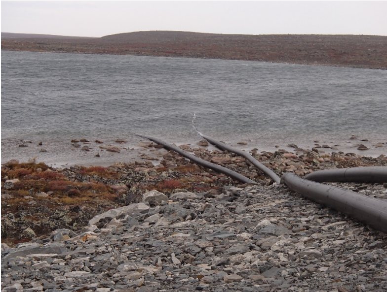
Photograph H4-1 Diffusers – Vault Diffuser
