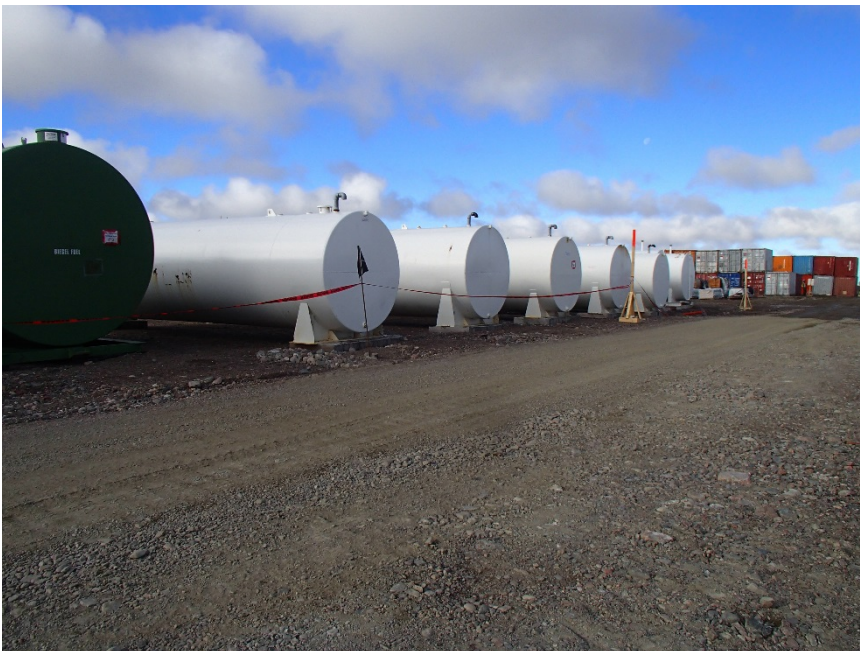
Photograph G4-2 Amaruq Tank Farm
