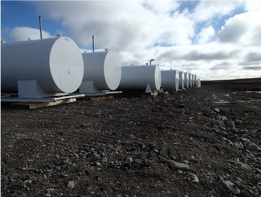
Photograph G4-5 Amaruq Tank Farm
