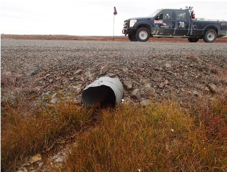
Photograph D1-6: PRC3 km 1+380
