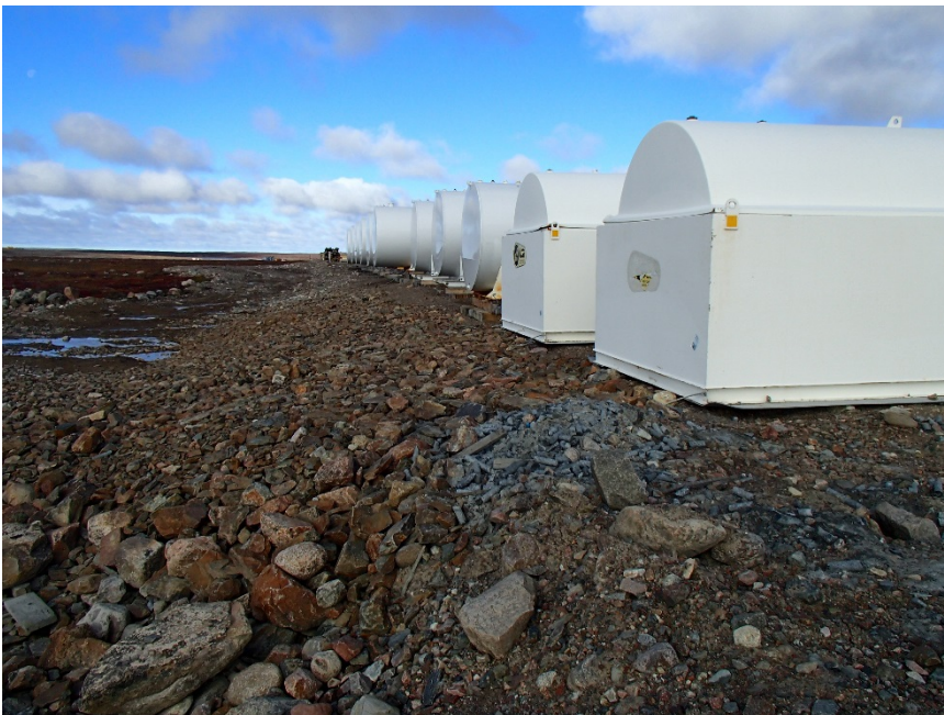
Photograph G4-4 Amaruq Tank Farm
