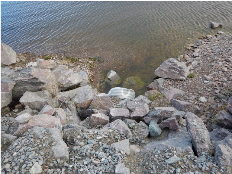
Photograph D1-2: PRC1 km 0+430
