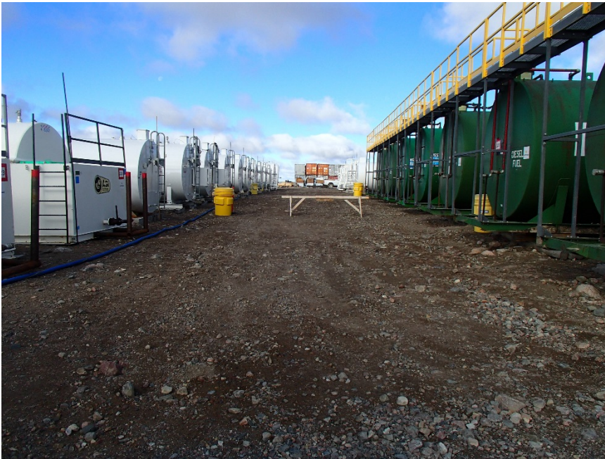
Photograph G4-3 Amaruq Tank Farm
