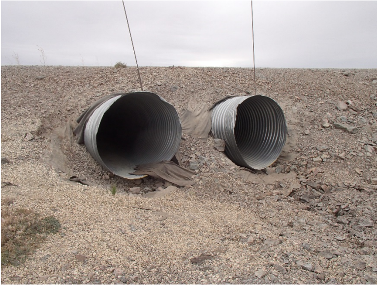
Photograph D1-11: PC-17A km 8+830
