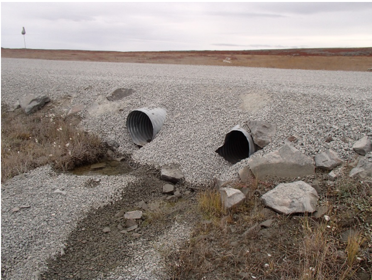
Photograph D1-38: PC-7A km 20+240
