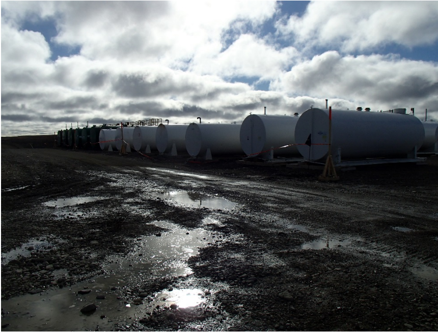
Photograph G4-7 Amaruq Tank Farm
