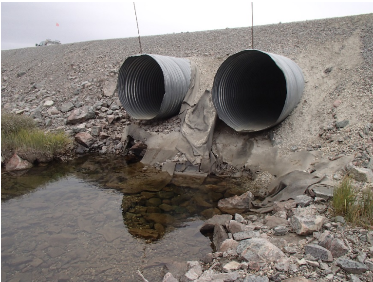
Photograph D1-12: PC-17A km 8+830
