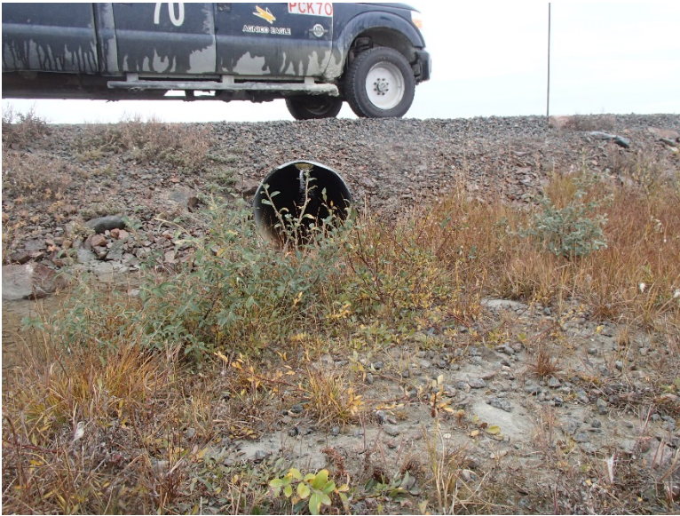
Photograph D1-5: PRC3 km 1+380
