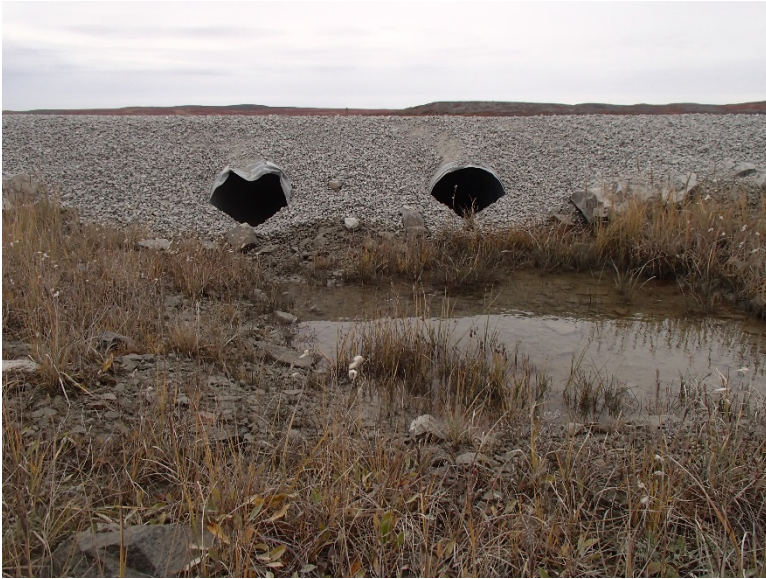
Photograph D1-37: PC-7A km 20+240
