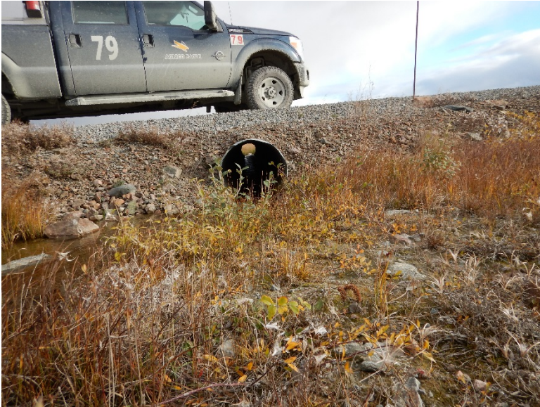
Photograph D1-5: PRC3 km 1+380
