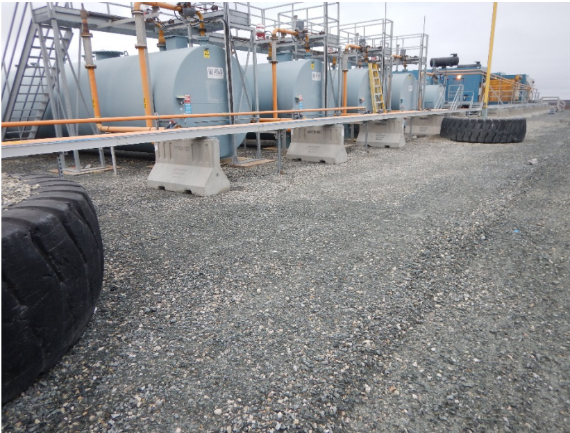
Photograph F3-3 Vault Tank Farm
