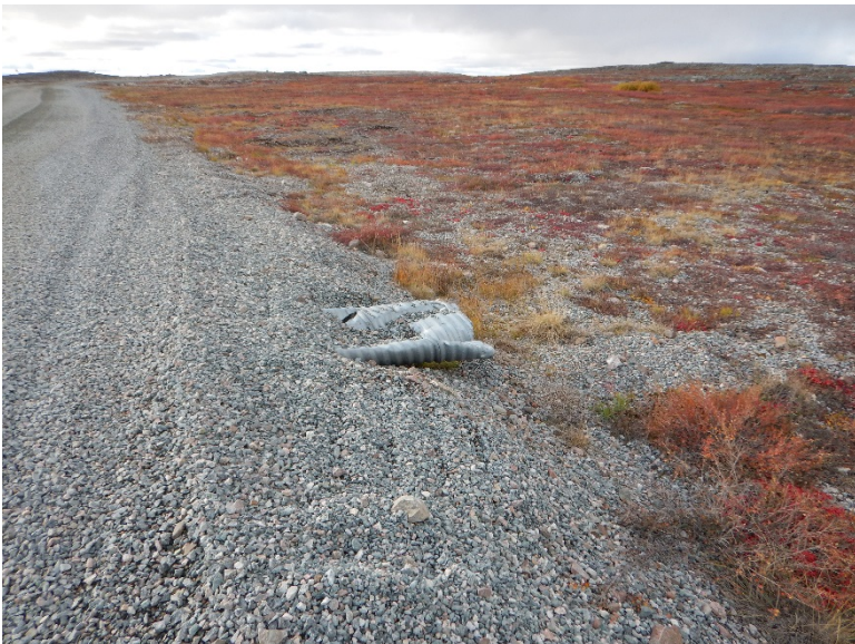
Photograph D1-8: R-00A km 2+550
