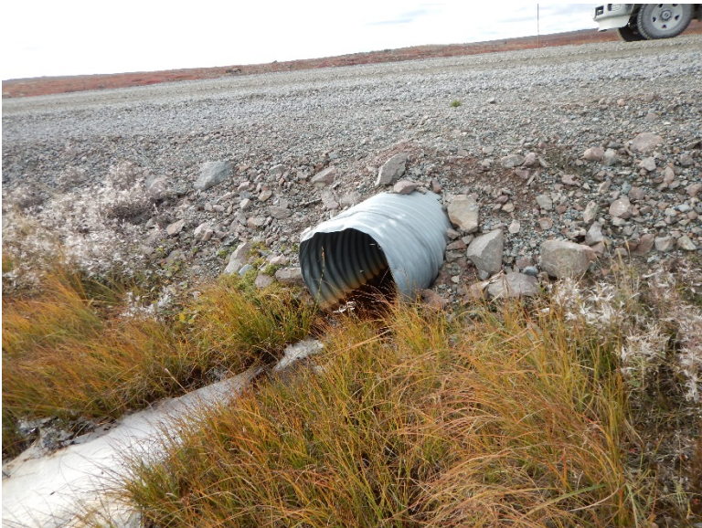
Photograph D1-6: PRC3 km 1+380
