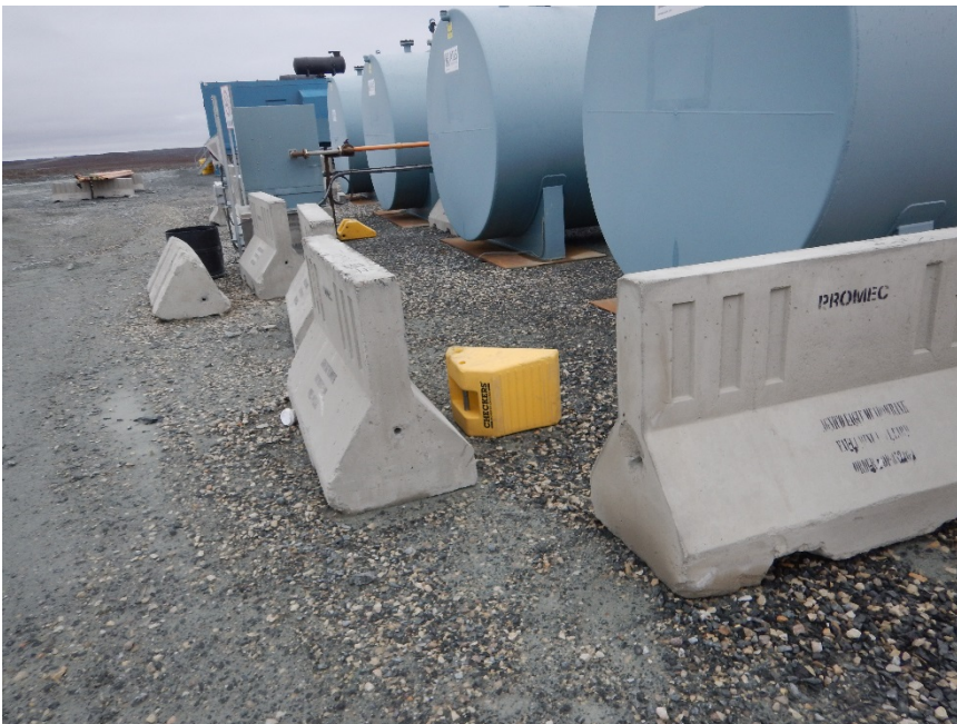
Photograph F3-2 Vault Tank Farm
