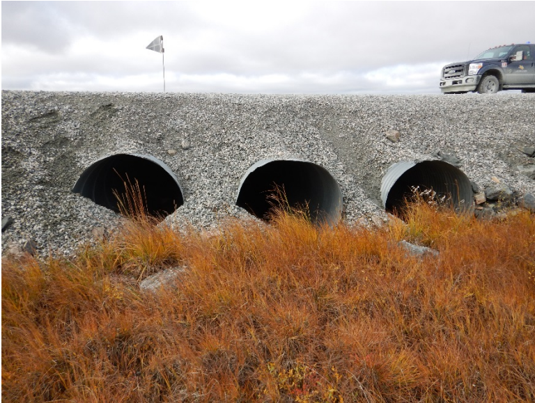
Photograph D1-59: R-18A km 80+950
