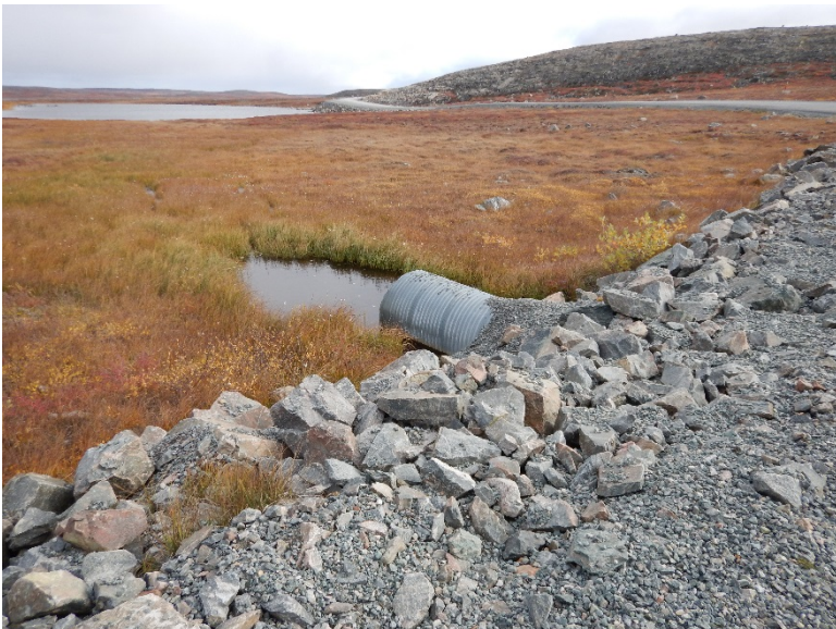
Photograph D1-34: R-05A km 15+745
