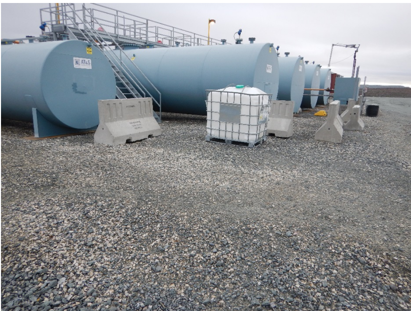
Photograph F3-4 Vault Tank Farm
