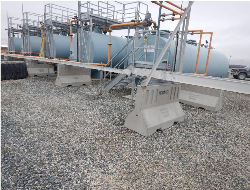
Photograph F3-1 Vault Tank Farm
