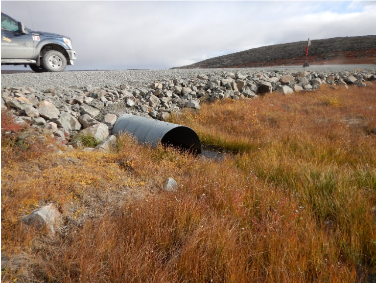
Photograph D1-33: R-05A km 15+745
