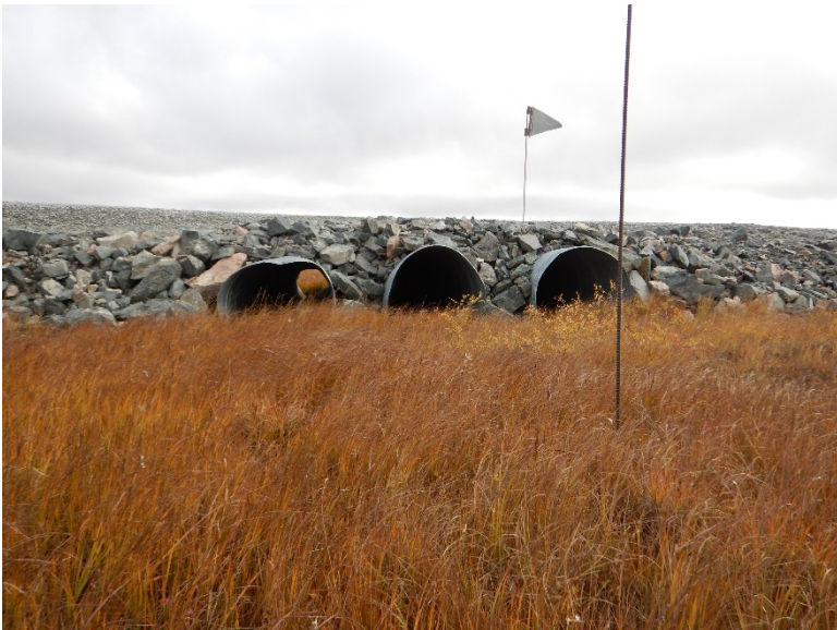
Photograph D1-60: R-18A km 80+950
