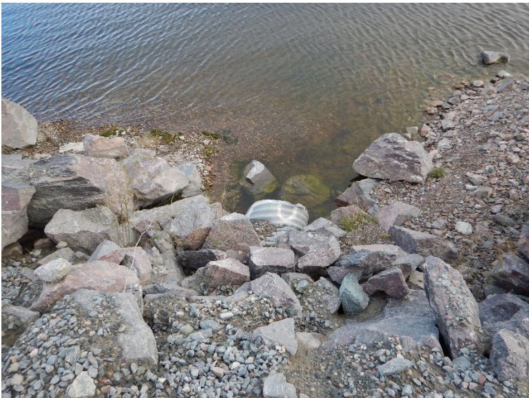
Photograph D1-2: PRC1 km 0+430
