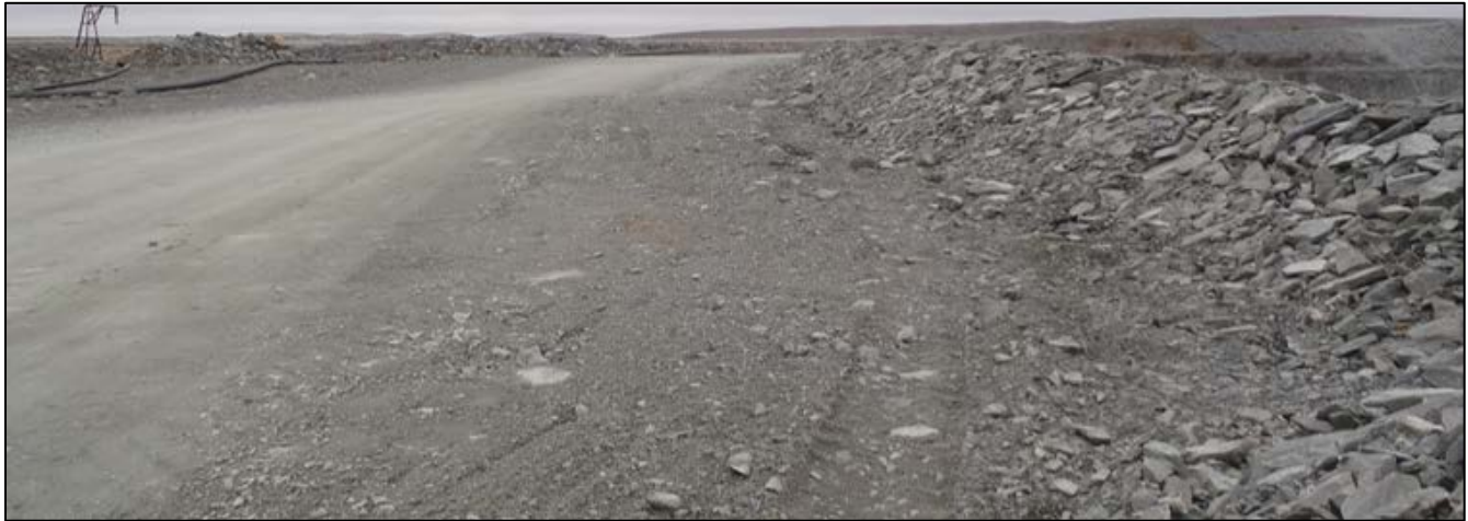
Photograph 8-17: Minor swale observed in ring road near 2015 inflow
