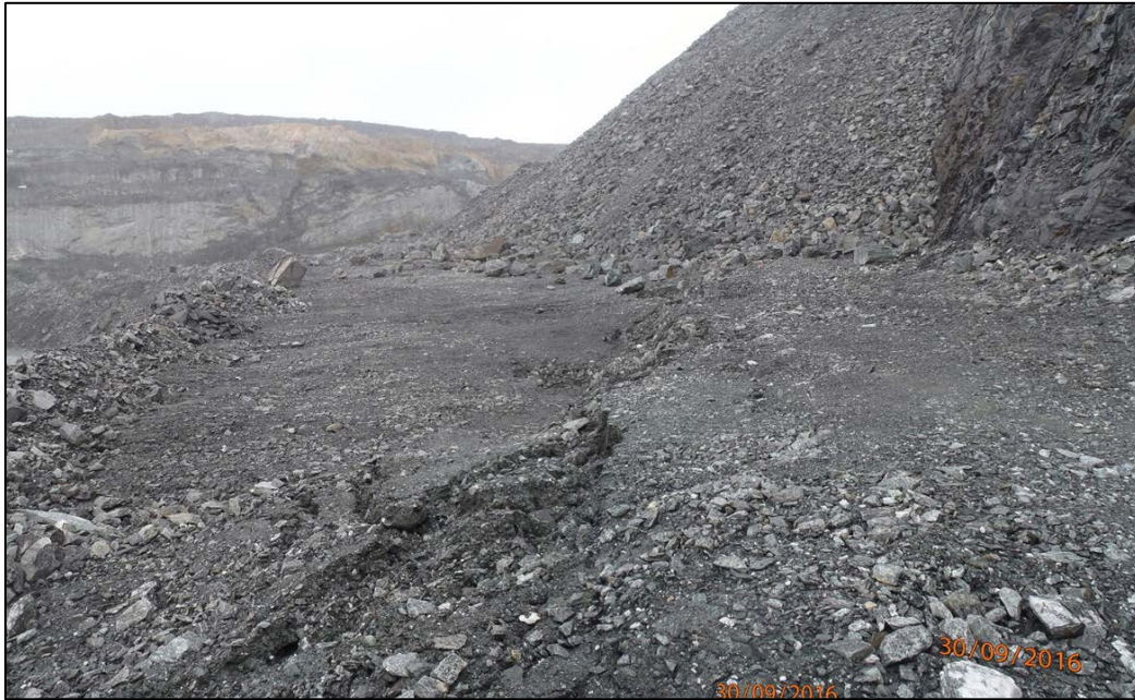
Photograph 5-3: Tension crack and settlement at eastern margin of lower platform, Pit D Dump (2016)
