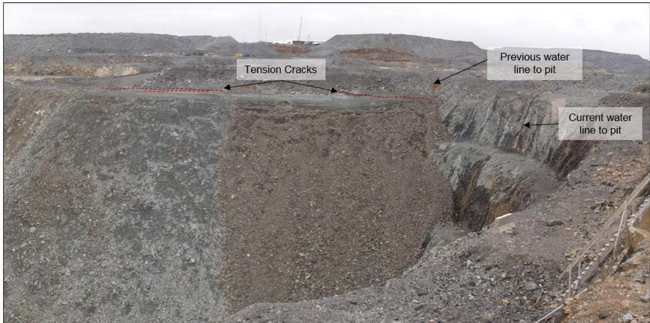
Figure 7-2: Location of tension cracks in Goose Pit dump platform (September 2016)
