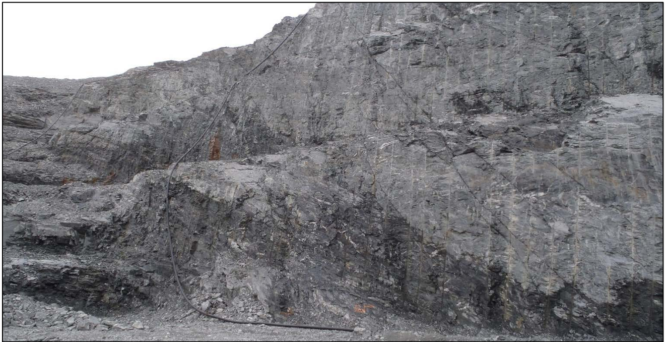
Photograph 8-22: Vault Pit north transition wall seepage along southeast dipping foliation planes
