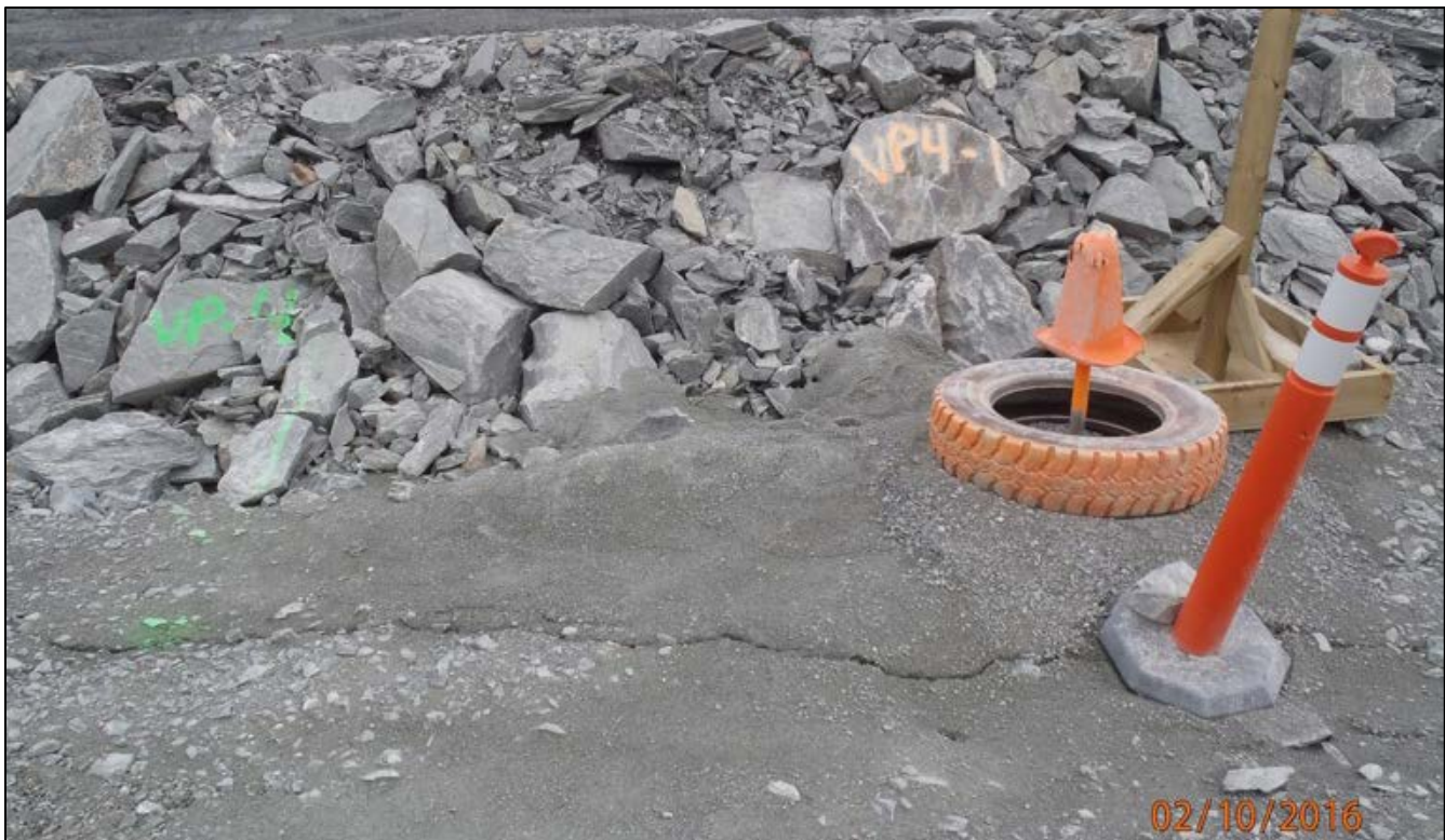
Photograph 8-16: Minor tension cracks noted in ring road near 2015 inflow
