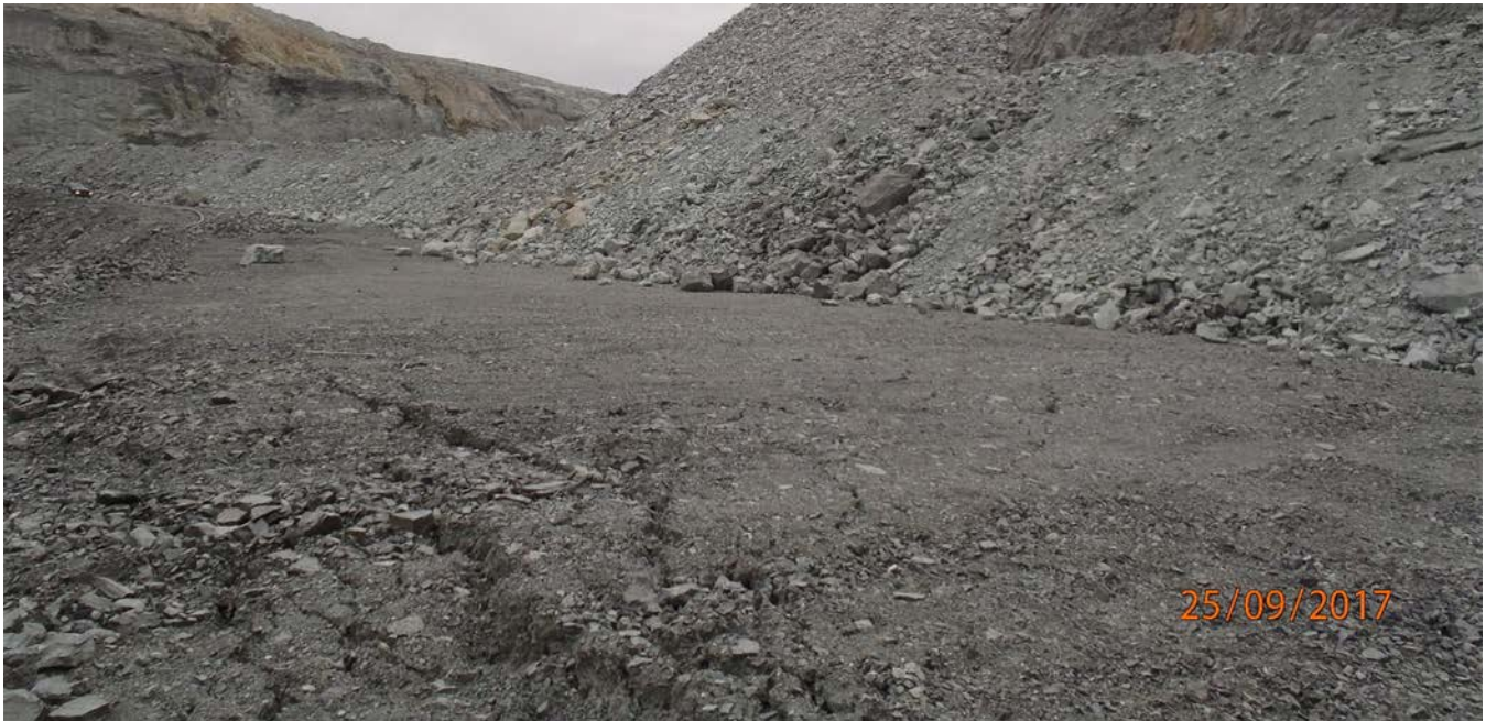
Photograph 5-3: D dump tension cracks at eastern margin of lower dump (2017)
