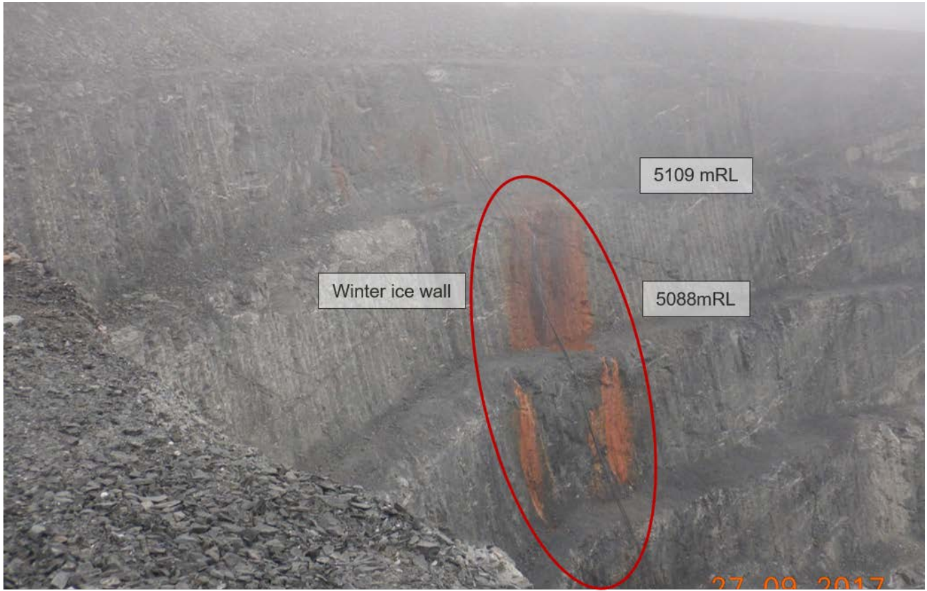
Photograph 8-10: Vault Pit seepage from southeast pit wall 5109 bench (2017)
