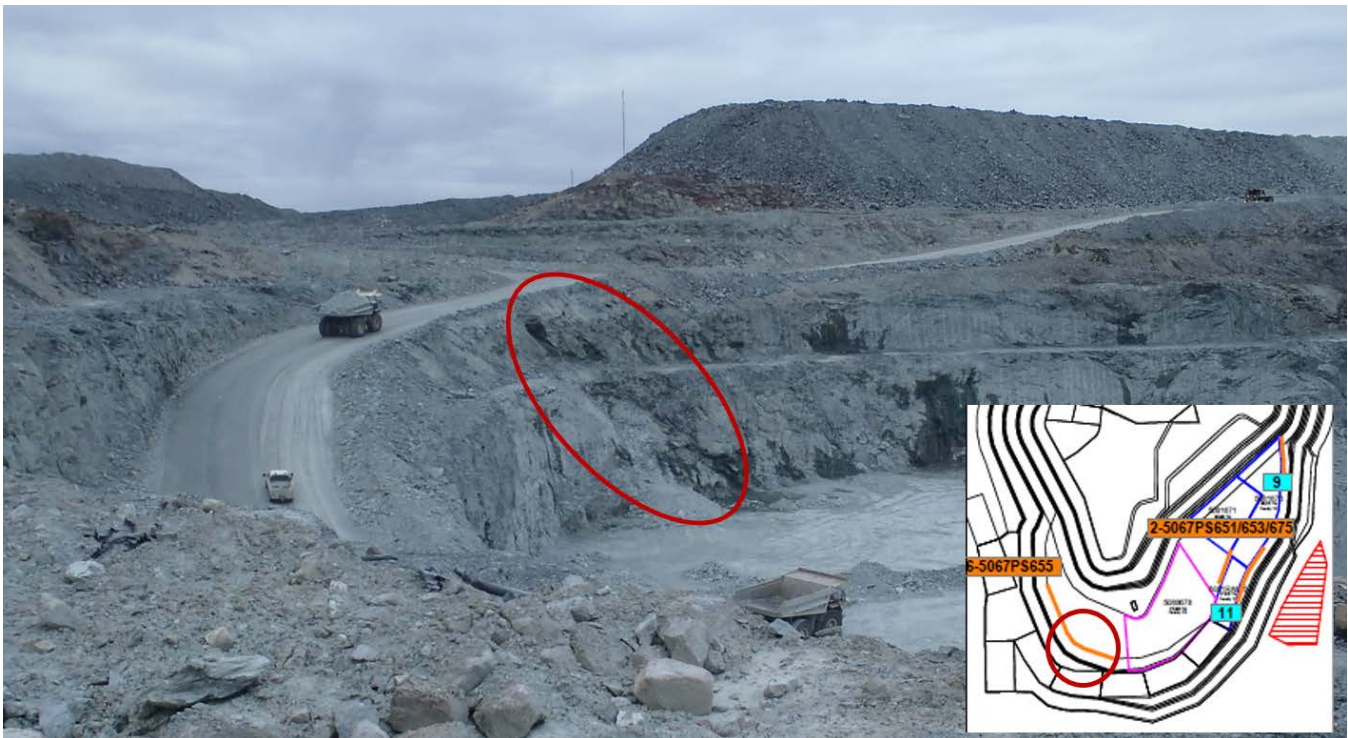
Photograph 6-7: Raveling of material below south ramp entry (south ramp wedge)
