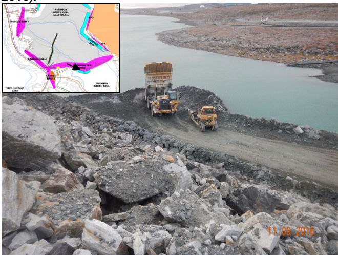
Figure 12: A haul truck dumps rockfill as the dozer stands by; at this point the buttress design has been changed to a width of 25m. Previously, the width was 15m between truck turnarounds. (September 11, 2016).
