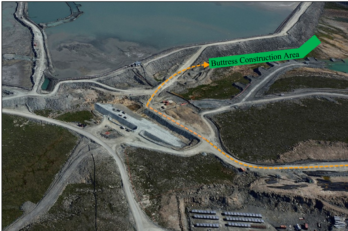
Figure 5: View of the plan for the access road for the SWD buttress (aerial photo from summer 2015 with access road plan added).
