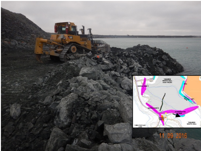
Figure 10: View of the dozer as it pushes rockfill to construct the buttress (September 11, 2016).
