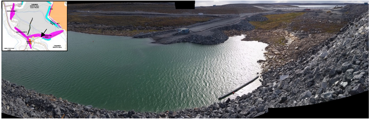
Figure 1: Photo of the Stormwater Dike downstream slope toe area prior to buttress construction looking south (September 1, 2016).
