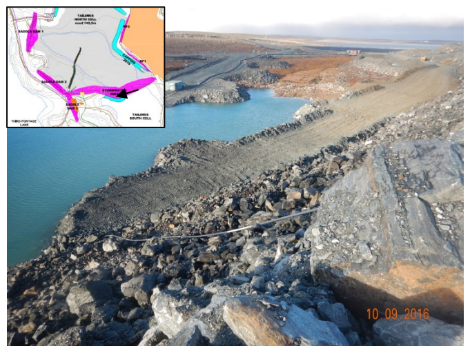
Figure 9: View of the buttress; note the turnaround area for the haul trucks (September 10, 2016).
