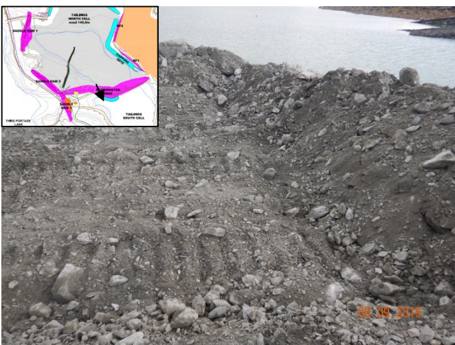
Figure 6: Close up view of the first lift of rockfill for the buttress (September 6, 2016).
