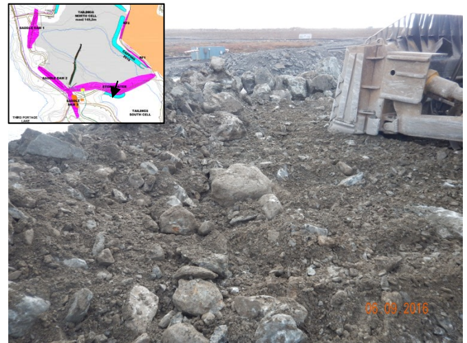
Figure 7: Close up view of the first lift of rockfill for the buttress (September 6, 2016).
