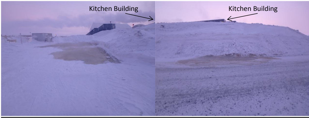
Photos 1-2- Seepage observed at the toe of the rockfill embankment, 2 locations (January 3 rd , 2016)
