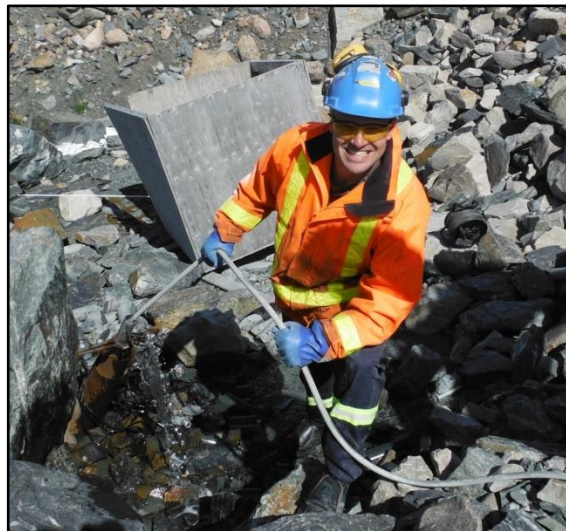
Melting 120 m of ice in MW-08-02 takes about 2 hours. Some water comes back up the well since ice is obstructing the well.
