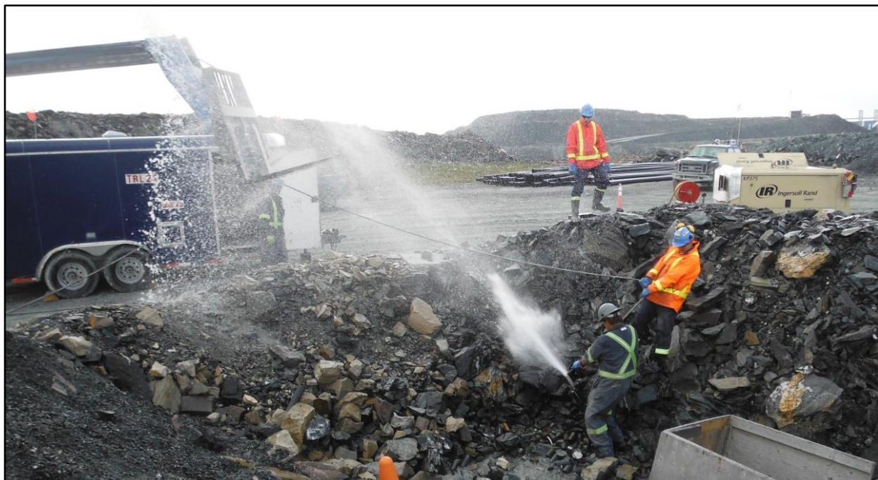
MW-08-02 was purged with compress air to remove the melted ice and the water added through the steaming operations. All the operations to free the well from ice together take an entire day. Despite the extensive purging, it is impossible to remove all trace of the operation from the well. The hose have to be extended on the ground and dirt end up going into the well. It is impossible to keep all material clean.
