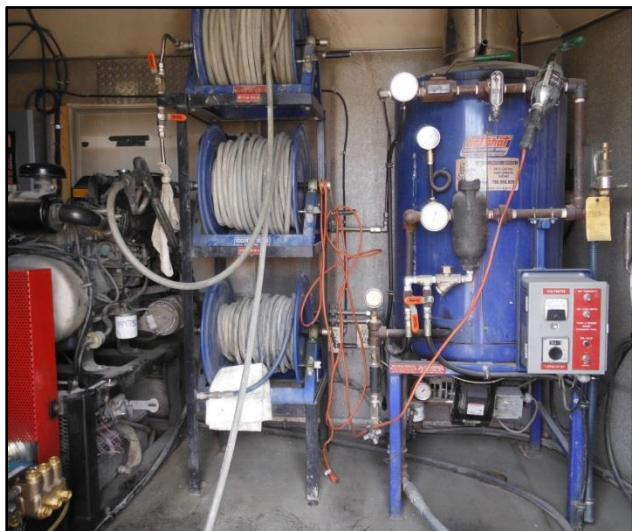
Since the heat traces on well MW-08-02 are damaged, the well is blocked with 120 m of ice. He ice is melted with a steamer used with 500 feet of hoses.
