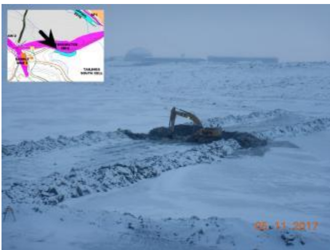
Photo 9: Close up view of a backhoe working on the first trench (November 5, 2017).
