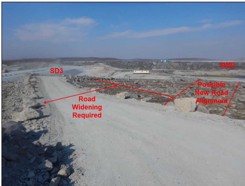
Figure 3: Road widening will be required on the Saddle Road as it turns toward Saddle Dam 3 since currently the road width is only enough for light vehicles. A new road could also be constructed to reduce the length of the hauling route, as seen on the right-hand side of the photo.
