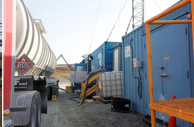
Photo 51: Overflow protection procedures
