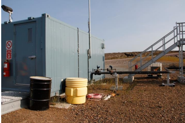
Photo 50: Refuelling station at the Baker Lake Fuel Tank Farm with Spill Containers in place
