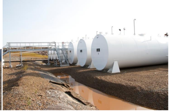
Photo 48: Baker Lake Aviation Fuel Tank Farm
