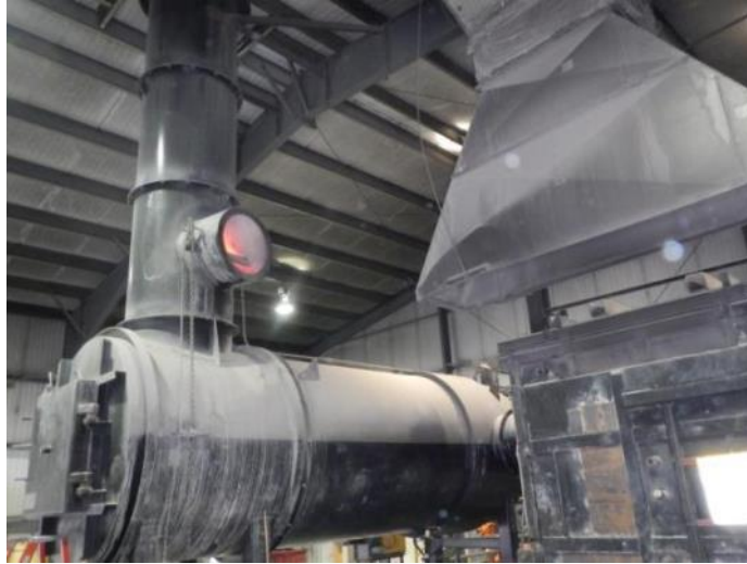
Photo 43: Incinerator at Meadowbank mine
