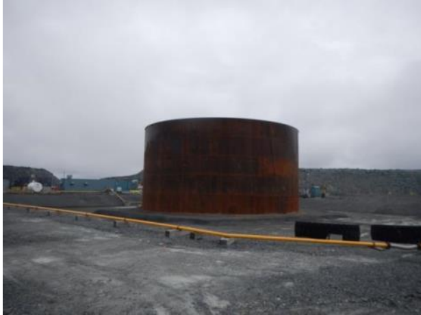
Photo 35: Meadowbank Fuel Tank Farm Facility
