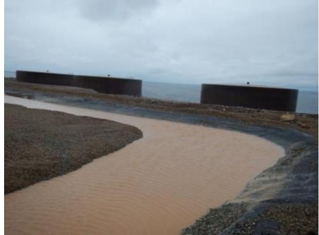
Photo 36: Water within the Baker Lake Fuel Tank Farm containment berm
