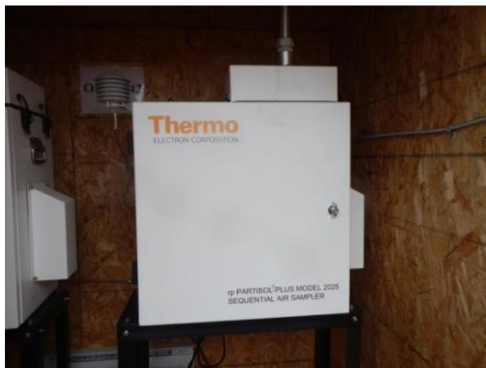
Photo 41: Air and partisol monitoring station near the emulsion station
