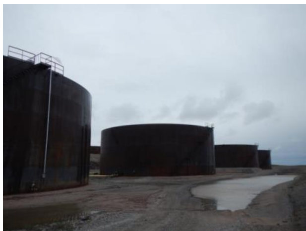
Photo 33: Baker Lake Fuel Tank Farm Facility
