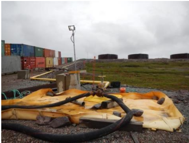
Photo 1: Secondary containment in place prior to fuel transfer at the Baker Lake laydown facility
