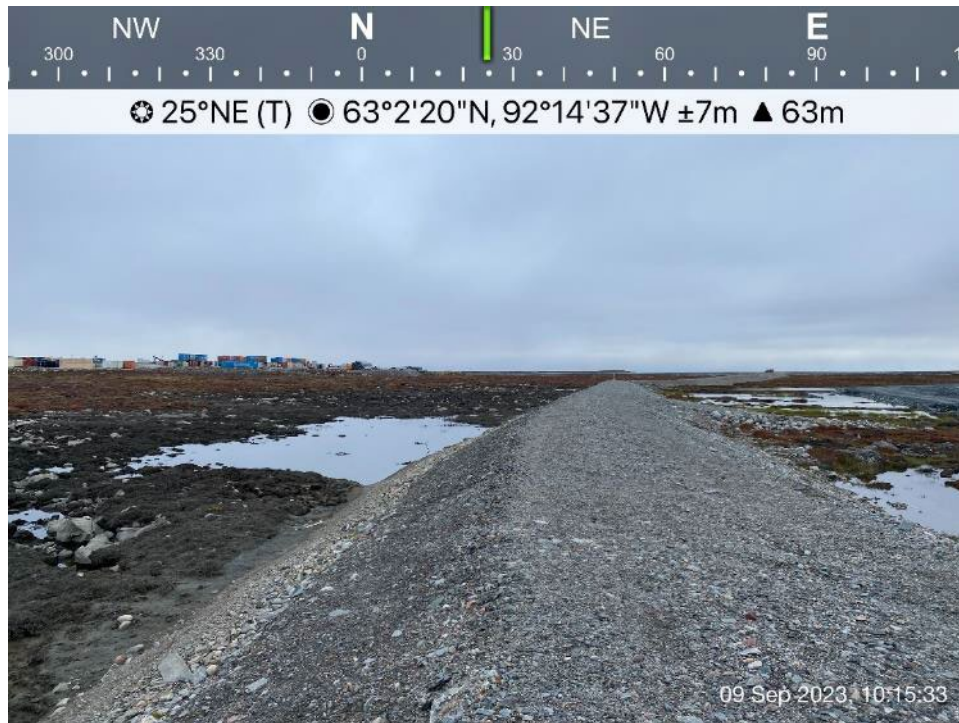
Berm 2 - Photo 14: Berm 2 - north section, ponded water on both sides.
