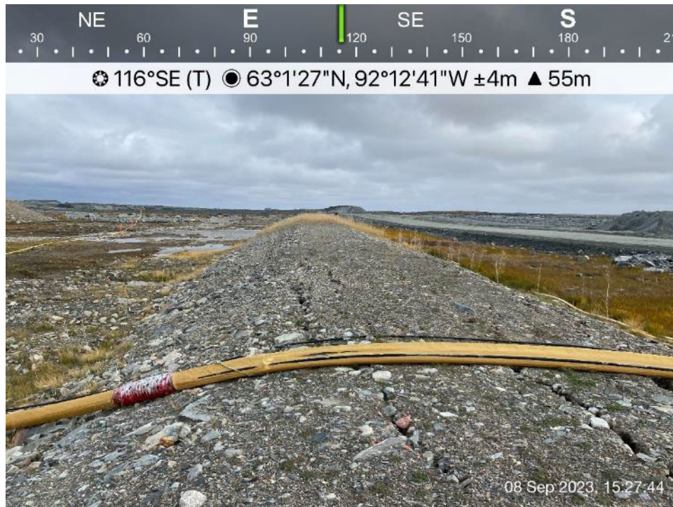
Berm 3 - Photo 19: Berm 3 - Berm crest, cracking observed along the crest.
