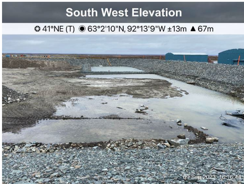
Landfarm - Photo 22: Landfarm - water collection pond and water ponding
