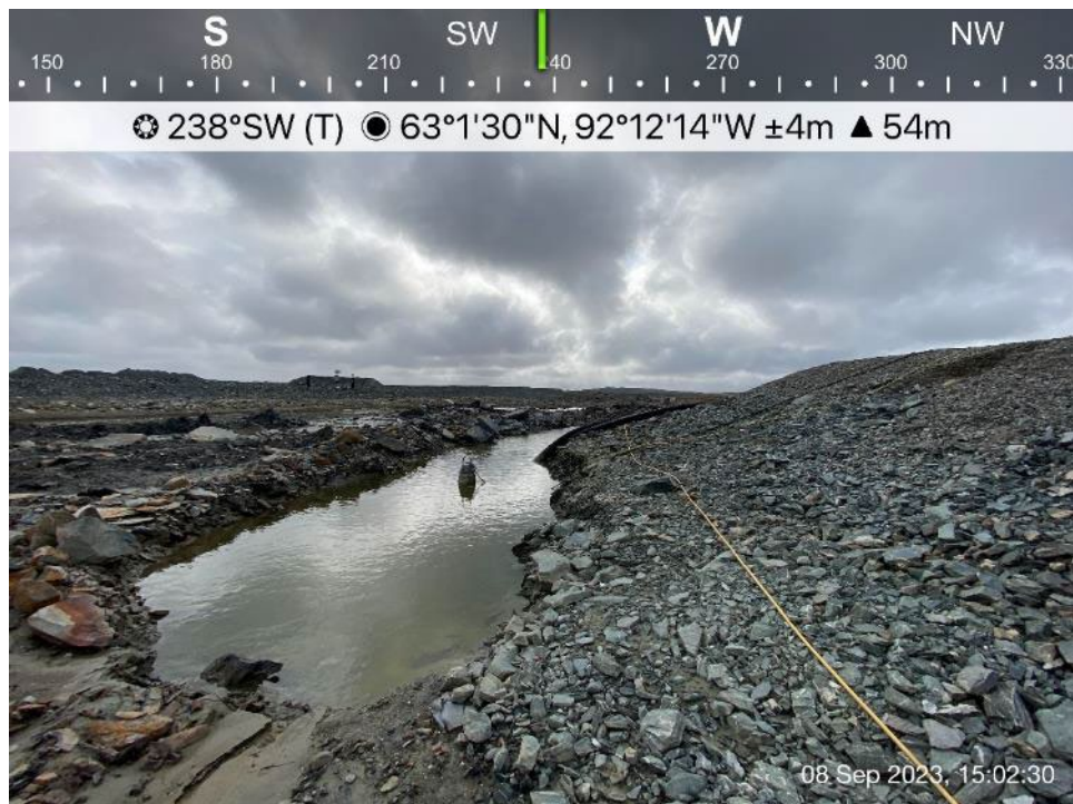
CP5 - Photo 6: CP5- Jetty and ditch around jetty, trash pump in the ditch to pump water out of CP5.
