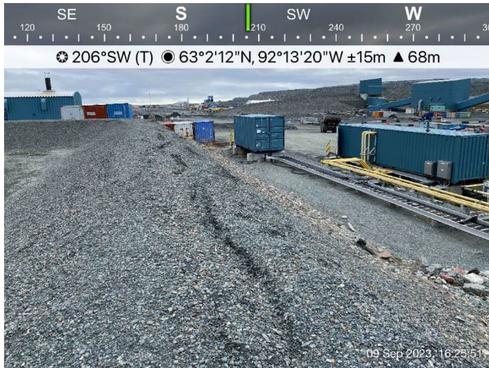
Industrial Fuel Tanks -Photo 25: Industrial Fuel Tanks - west side berm, looking southwest.
