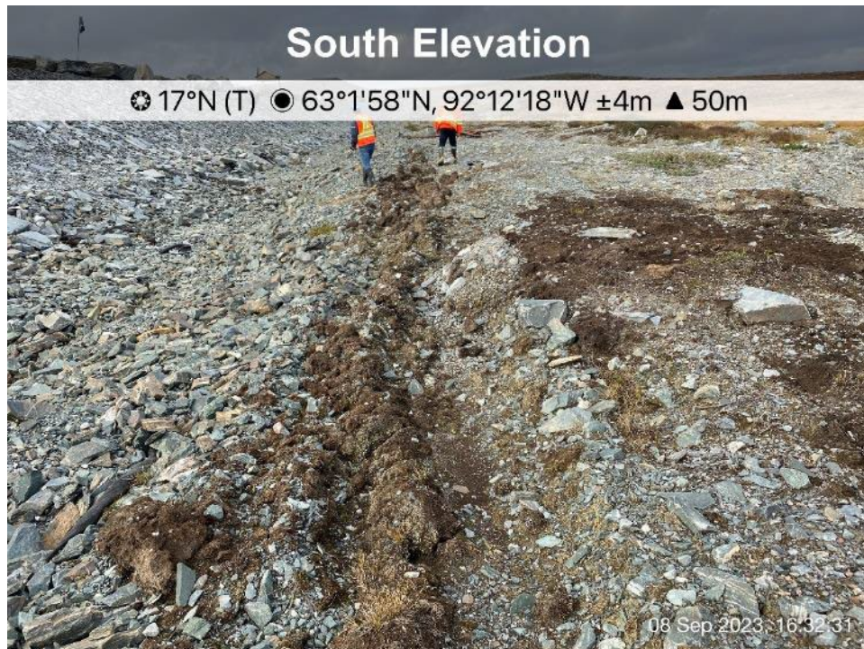
D-CP1 - Photo 13: Dike D-CP1: Dike downstream runoff/seepage collection north channel - thaw subsidence on east channel shoulder.
