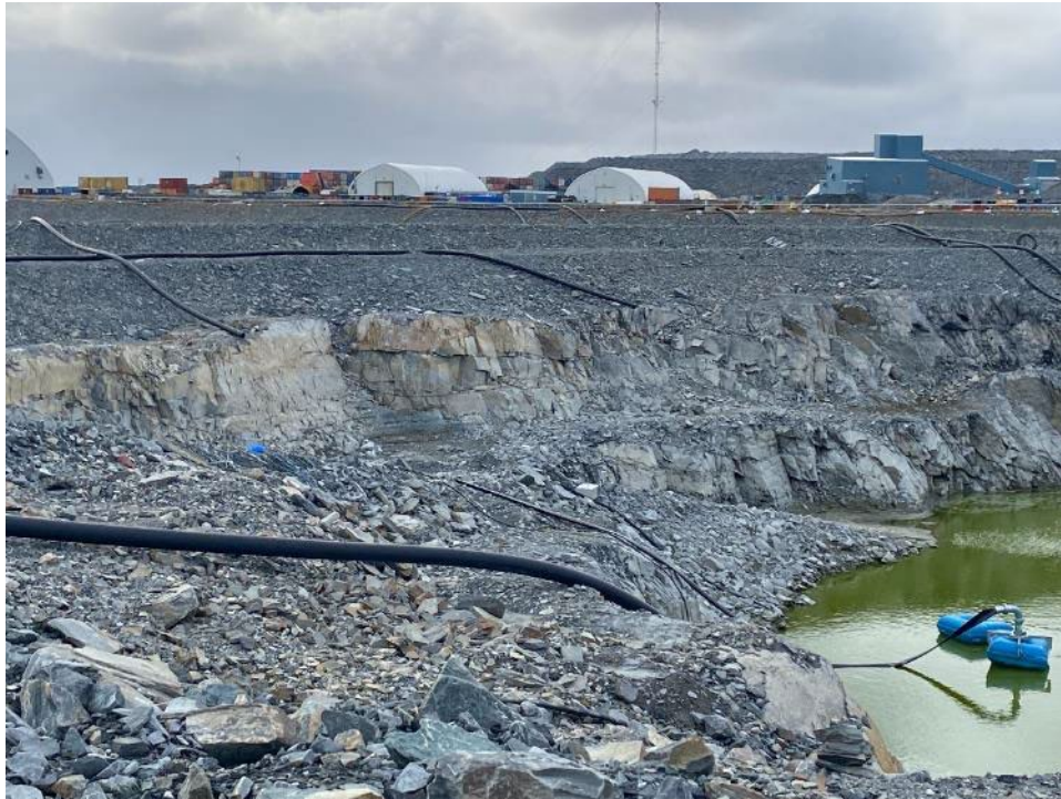
SP1 - Photo 3: SP1 Saline Pond - Perimeter berm side slope and bedrock side wall.
