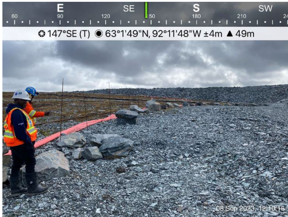
CP6 - Photo 10: CP6 East side perimeter, thaw settlement observed.
