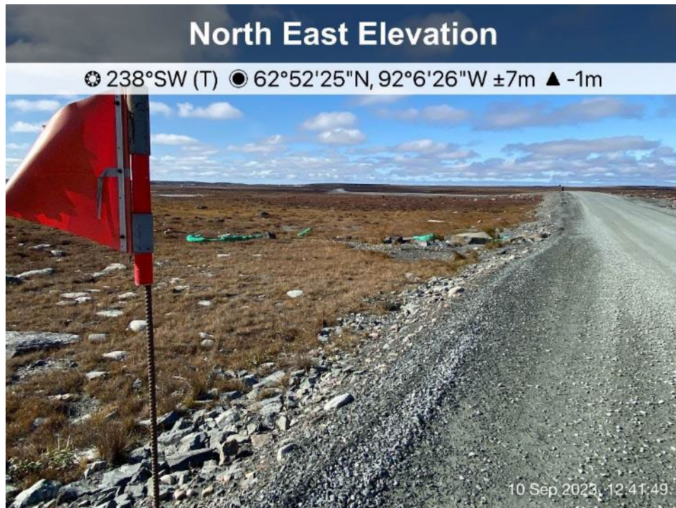
AWAR Road/Culvert - Photo 21: KM 8.8 - No culvert installed, water overflows the road during freshet.
