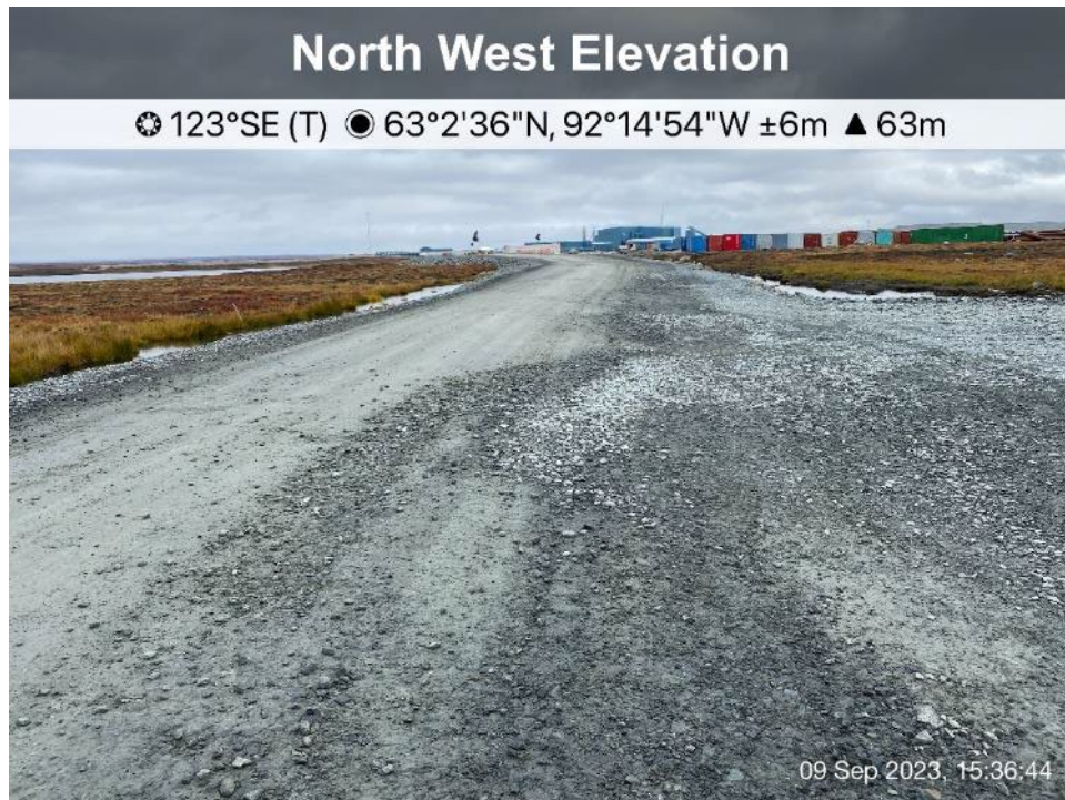
Site Road - Photo 1: Site Road - Road to Emulsion AN Pad and storage area.
