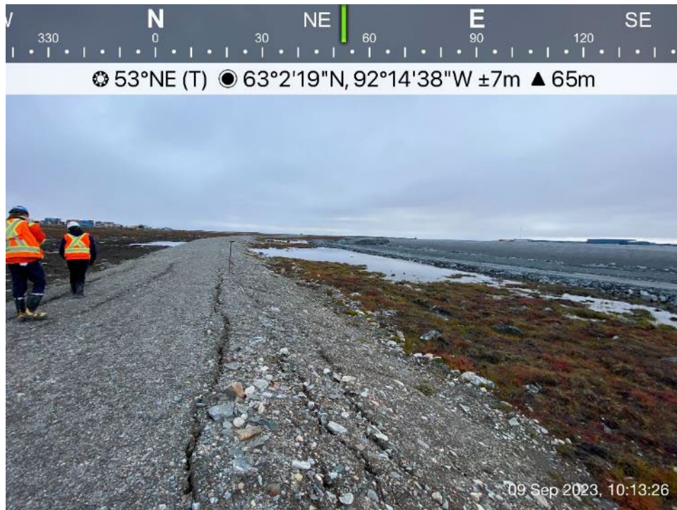
Berm 2 - Photo 13: Berm 2 - ponded water on both sides, cracking observed on slope and crest.
