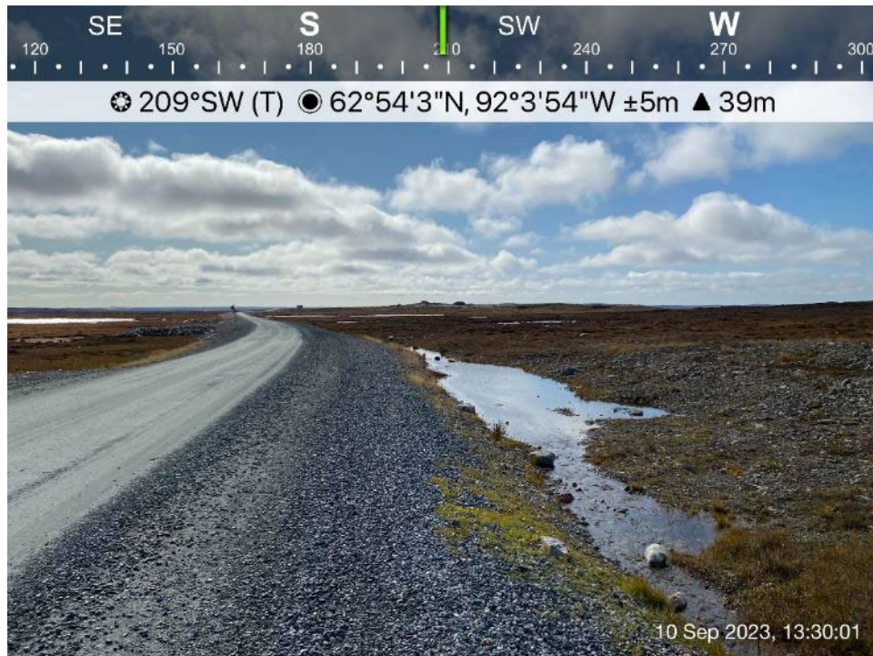
AWAR Road/Culvert - Photo 33: KM 12.6 - No culvert installed, poor drainage condition, no sign of water flow.
