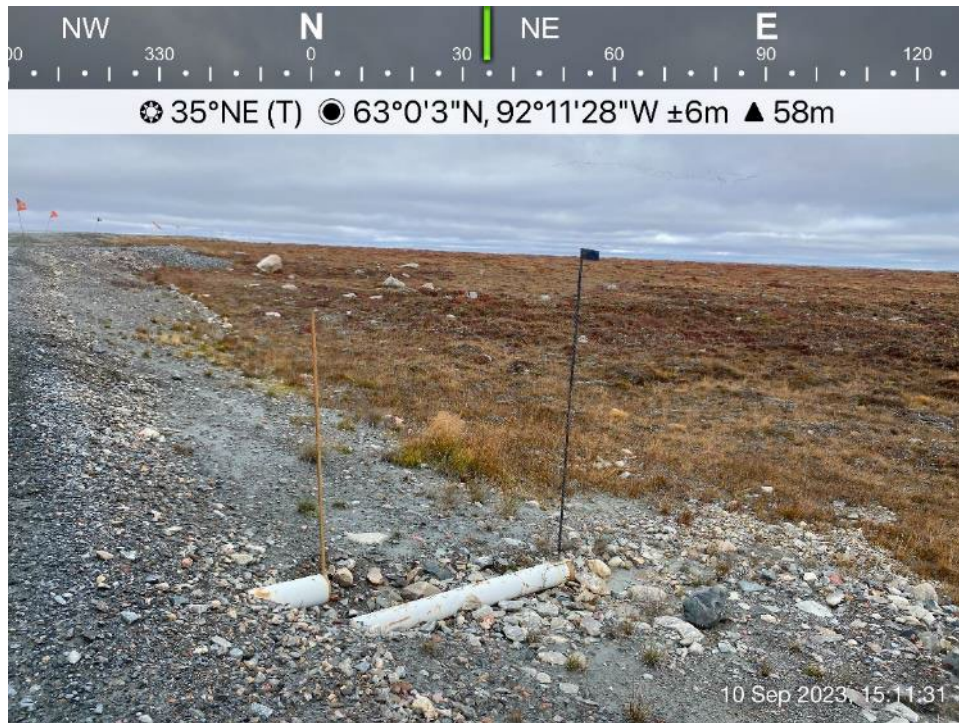
AWAR Road/Culvert - Photo 63: Culvert KM 26.8 - steel pipe as culvert, inlet is above water level.
