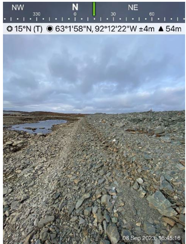
D-CP1 - Photo 2: Dike D-CP1: Upstream face - some wave erosion evident from 2019/2020 high water level event, no change from previous years.
