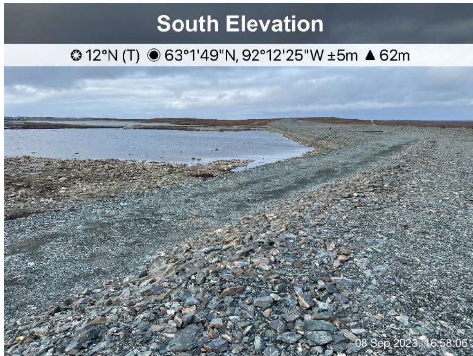
D-CP1 - Photo 1: Dike D-CP1: Upstream face - some wave erosion evident from 2019/2020 high water level event, no change from previous years.
