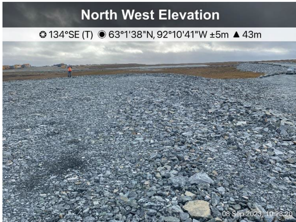
CP2 Thermal Berm - Photo 5: CP2 Thermal Berm - crest, east end, minor settlement observed, no cracking.
