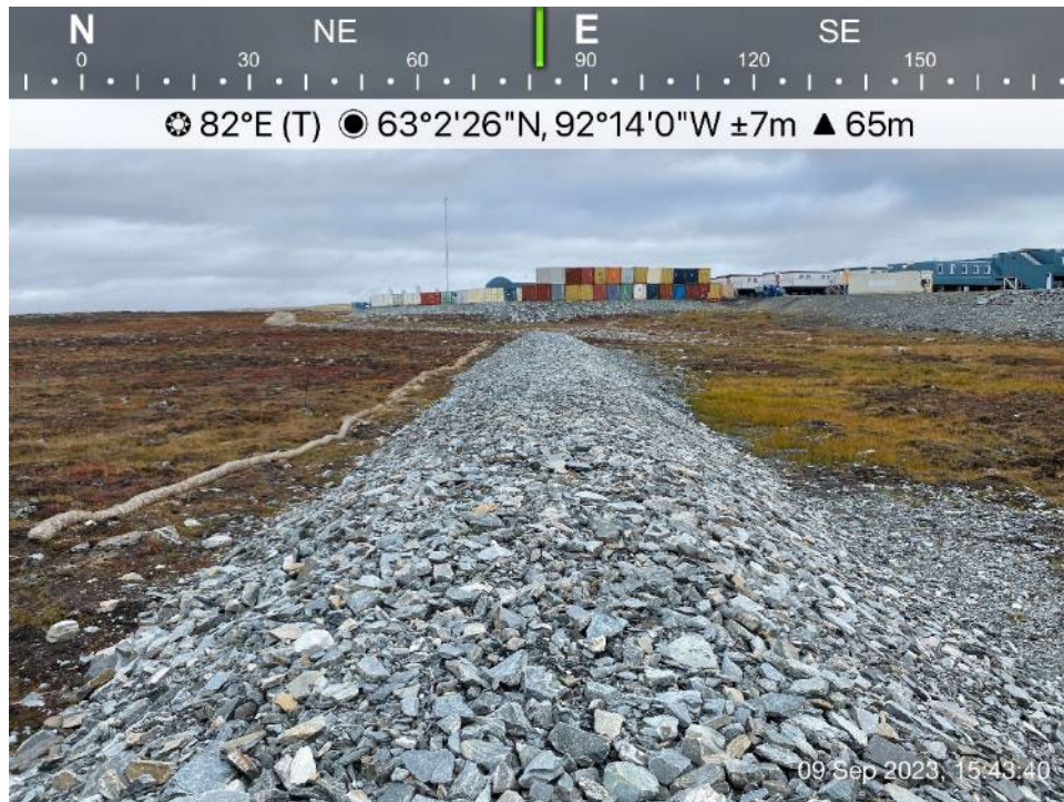
Channel 2 Berm - Photo 20: Channel 2 Berm - Overview of the new constructed Channel 2 Berm.
