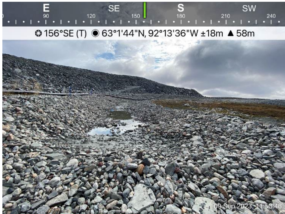
Channel 4 - Photo 13: Channel 4 - Settlement in base of channel resulting in minor ponding.
