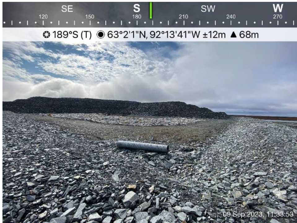
Landfill - Photo 12: WRSF1 Landfill - drainage well (to be installed for water management).
