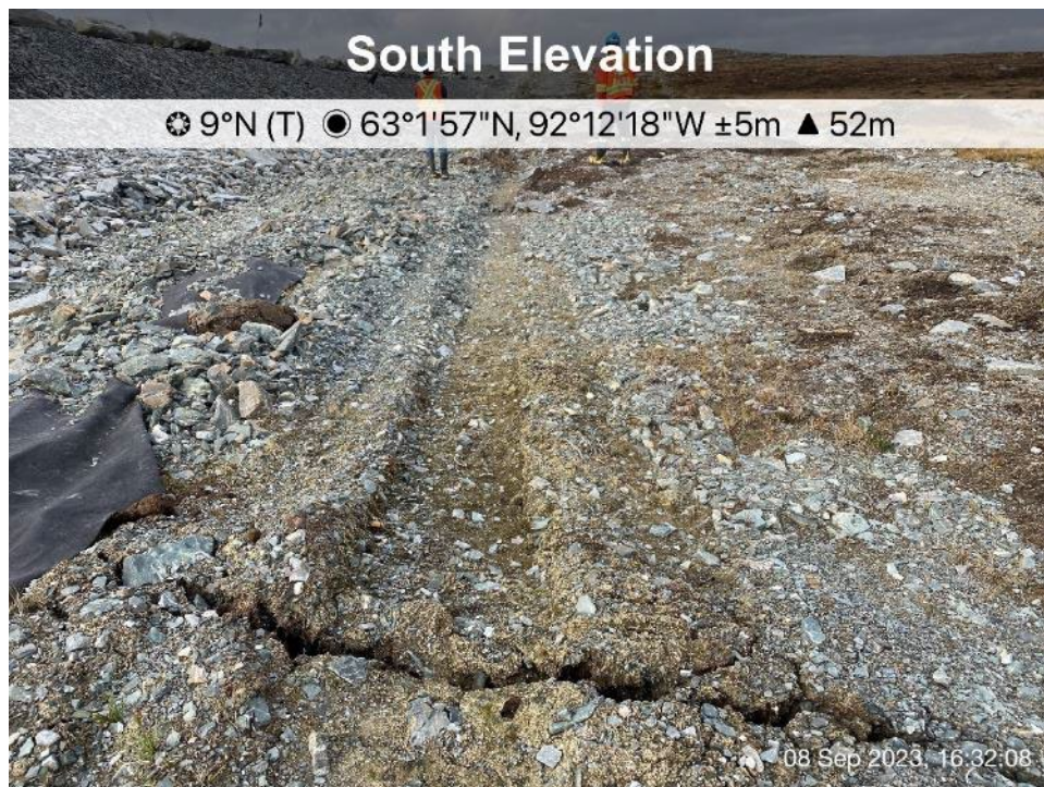
D-CP1 - Photo 12: Dike D-CP1: Dike downstream runoff/seepage collection north channel - cracking on east channel shoulder.
