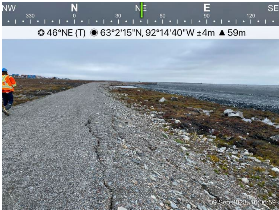
Berm 2 - Photo 12: Berm 2 - Berm 2 middle portion, slope and crest, cracking observed on upstream slope.
