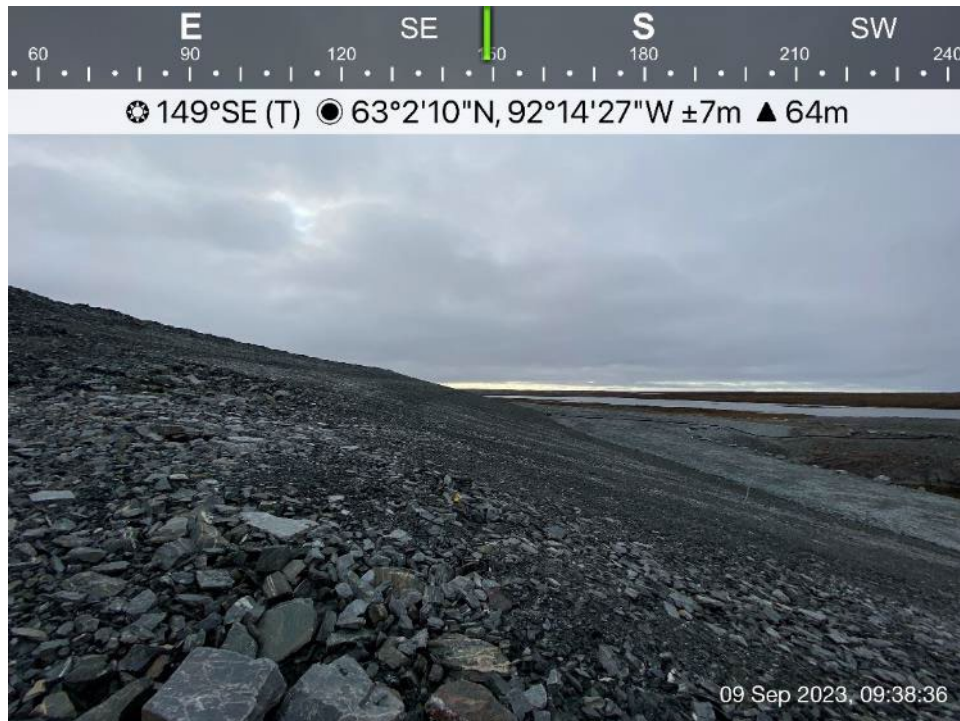
TFS - Photo 5: TFS - Rockfill cover slope along west side of Cell 1, looking southeast.
