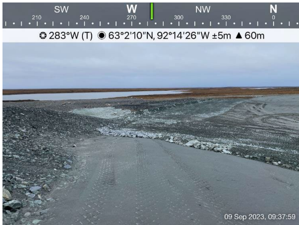
TSF - Photo 4: TSF - Rockfill cover of tailings along west side of Cell 2, looking west.
