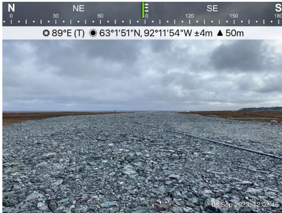
CP6 - Photo 7: CP6 Thermal Berm, looking east, crest, thaw settlement observed at various areas.
