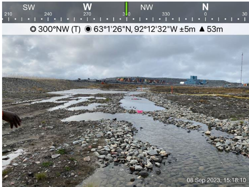
Channel 5 - Photo 12: Channel 5 - Upper section of Channel 5, ponded water observed due to thaw subsidence, looking northwest.
