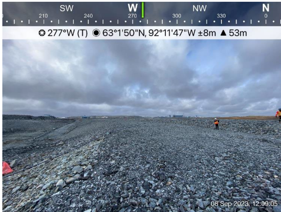
CP6 - Photo 8: CP6 Thermal Berm, looking west, berm crest and upstream slope, CP6 on the left.
