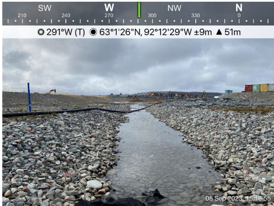
Channel 5 - Photo 11: Channel 5 - Middle section of Channel 5, ponded water observed due to thaw subsidence, looking west.
