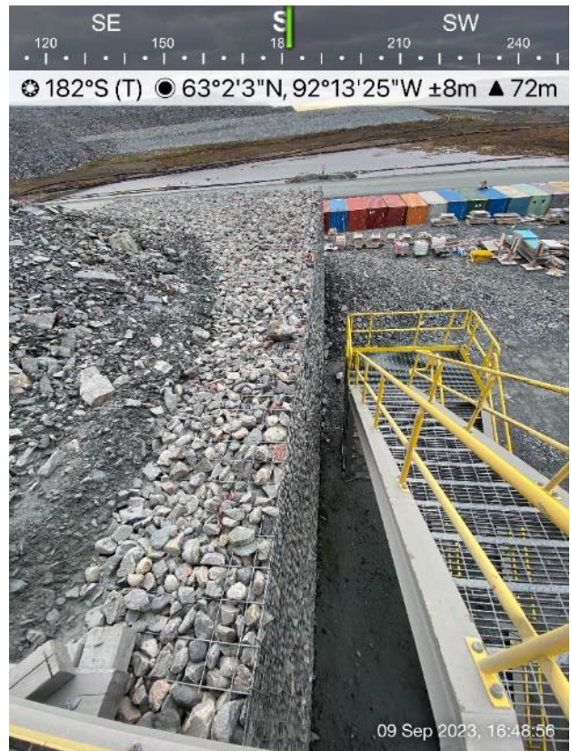
Crusher Pad - Photo 4: Crusher Pad - MSE retaining wall on the northwest corner, looking south.
