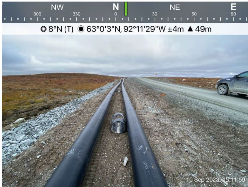
AWAR Road/Culvert - Photo 64: Culvert KM 26.8 - steel pipe as culvert, outlet was buried during the waterline project construction.
