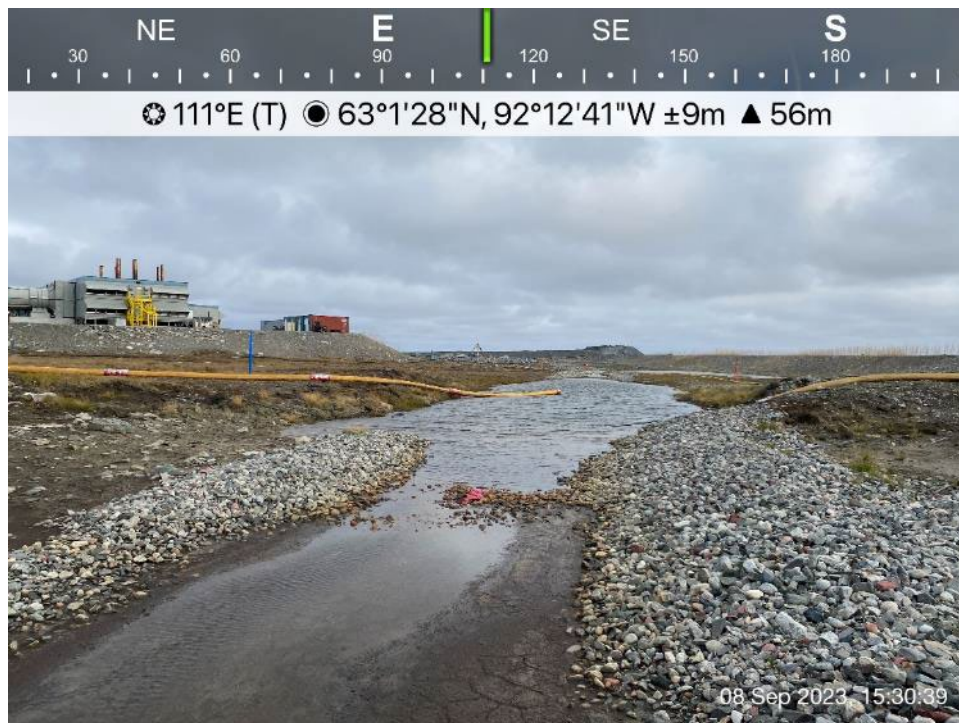
Channel 5 - Photo 14: Channel 5 - Upper section of Channel 5, significant subsidence and cracking along slopes with riprap settled below water level in channel, filled with sedimentation from surface erosion.
