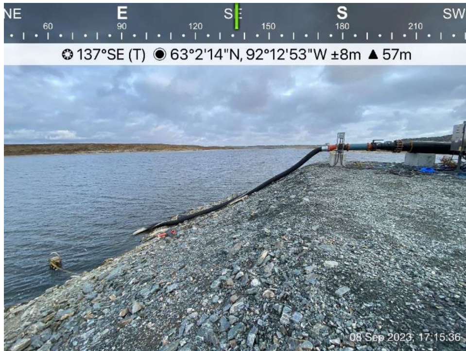
D-CP1 - Photo 18: Dike D-CP1: Jetty 1 water intake - minor erosion, no change from previous years.
