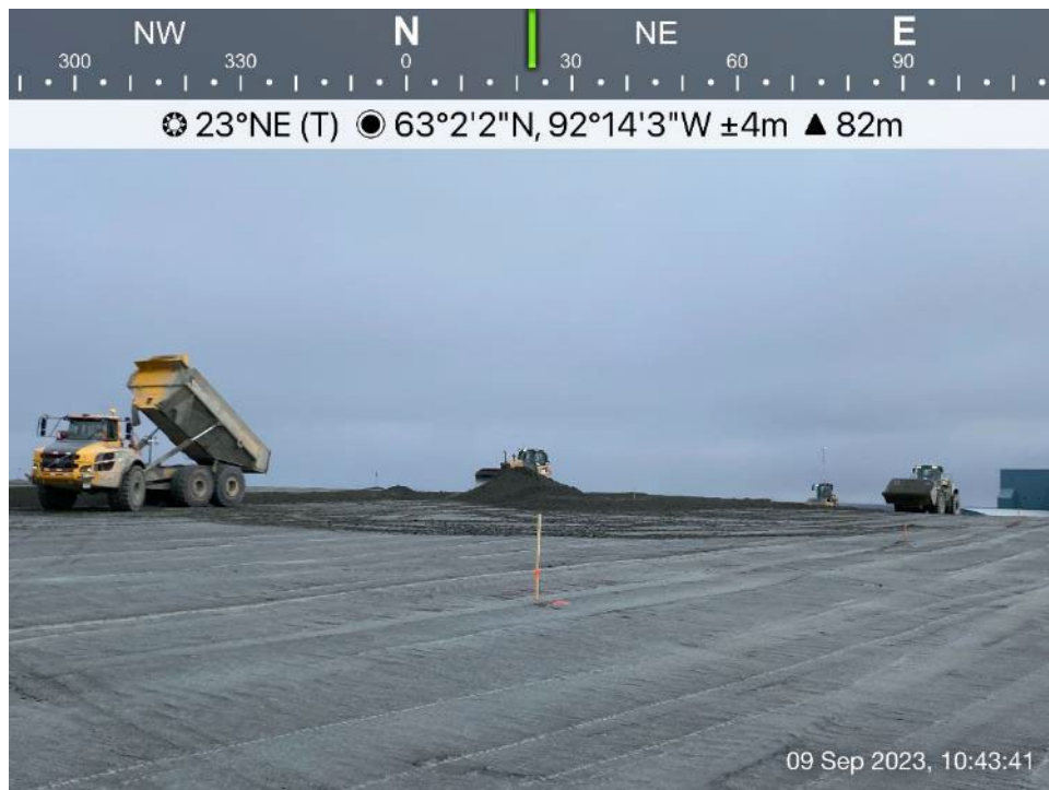
TFS - Photo 6: TFS - dumping, spreading and compacting of the tailings in Cell 1.
