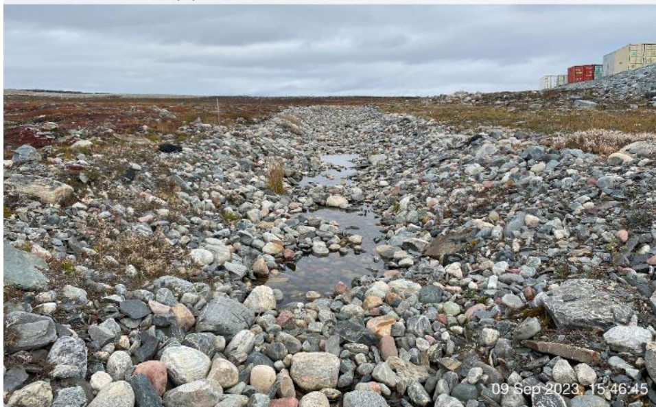
Channel 2 - Photo 6: Channel 2 -Middle section, minor water ponding observed at the base of channel due to thaw subsidence.
