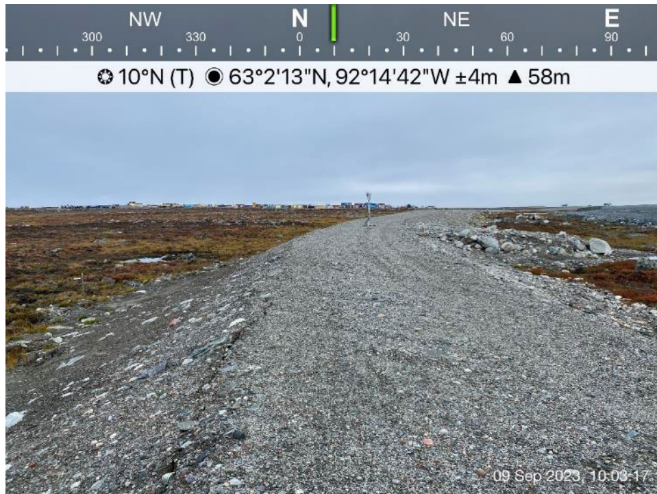
Berm 2 - Photo 10: Berm 2 - Berm 2 south portion, slope and crest, cracking observed on downstream slope.
