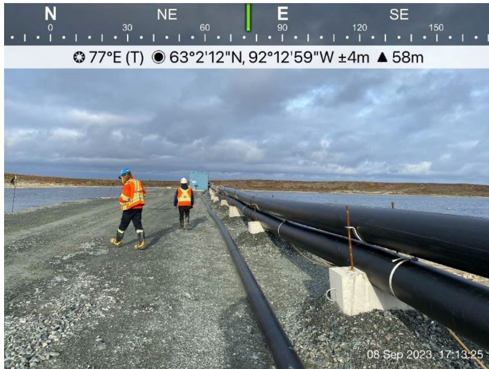
D-CP1 - Photo 17: Dike D-CP1: Pipelines on Jetty 1.
