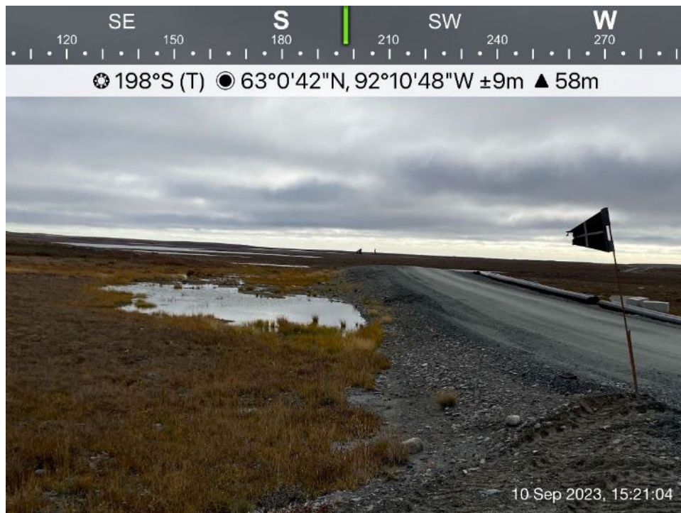
AWAR Road/Culvert - Photo 68: KM 28.7 - No culvert installed, ponded water upstream.
