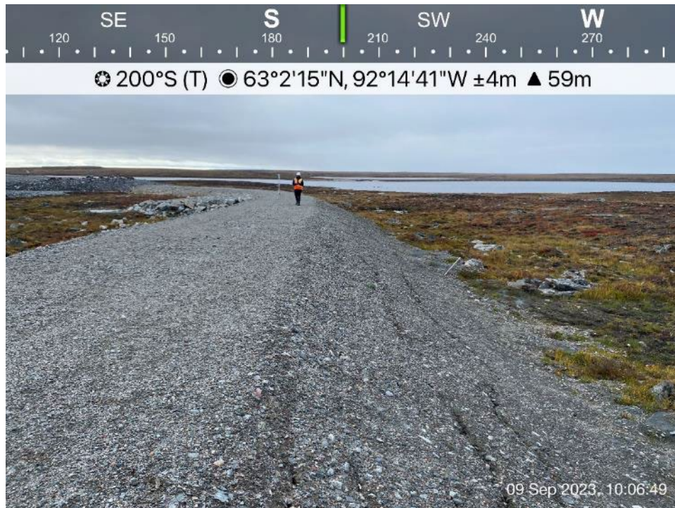
Berm 2 - Photo 11: Berm 2 - Berm 2 middle portion, slope and crest, cracking observed on downstream slope.
