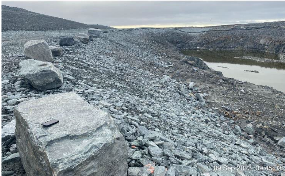
CP3 - Photo 2: CP3- waste rock cover placed between TSF toe and CP3 as thermal protection.
