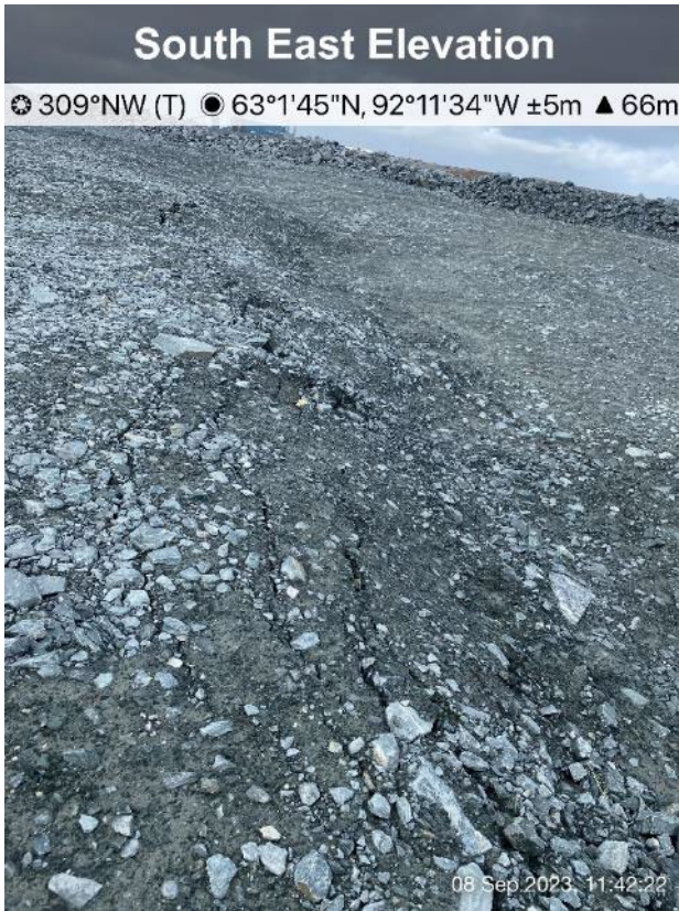
WRSF3- Photo 3: WRSF 3 - settlement and cracking observed on Bench 72 m.
