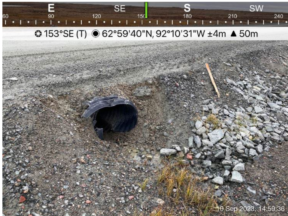
AWAR Road/Culvert - Photo 57: Culvert KM 25.8 - HDPE corrugated culvert - sign of deformation observed.
