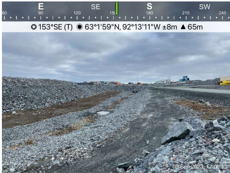
Channel 7 - Photo 15: Channel 7 - Upper reach and middle section of Channel 7, minor water ponding and thaw subsidence.
