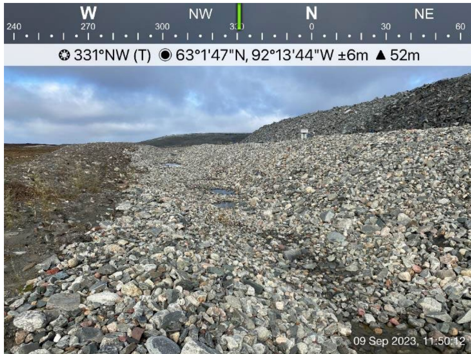
Channel 4 - Photo 12: Channel 4 - Settlement in base of channel resulting in minor ponding, subsidence in downstream slope of channel.
