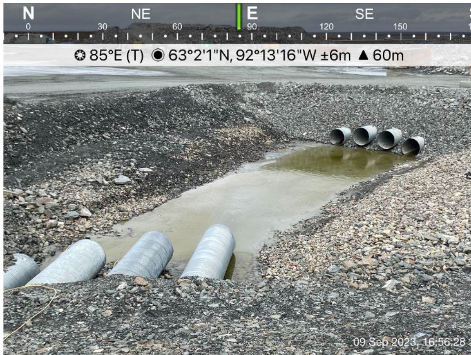
Channel 1 - Photo 3: Channel 1 - Channel length between crusher ramp and ore pad access, looking east.
