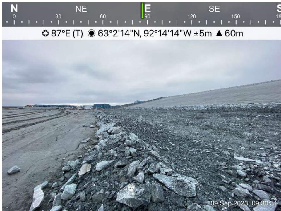
TSF - Photo 2: TSF - Rockfill berm constructed between Cell 1 and Cell 2 tie-in to reduce the surface erosion of north slope of Cell 1.
