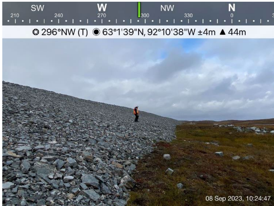
CP2 Thermal Berm - Photo 7: CP2 Thermal Berm - downstream slide slope, minor deformation observed at east end, no stability concern.
