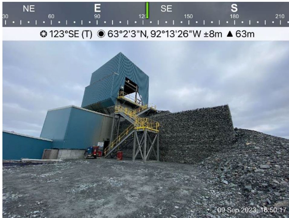
Crusher Pad - Photo 6: Crusher Pad - Overview of MSE retaining wall and crusher building - northwest side, looking southeast.
