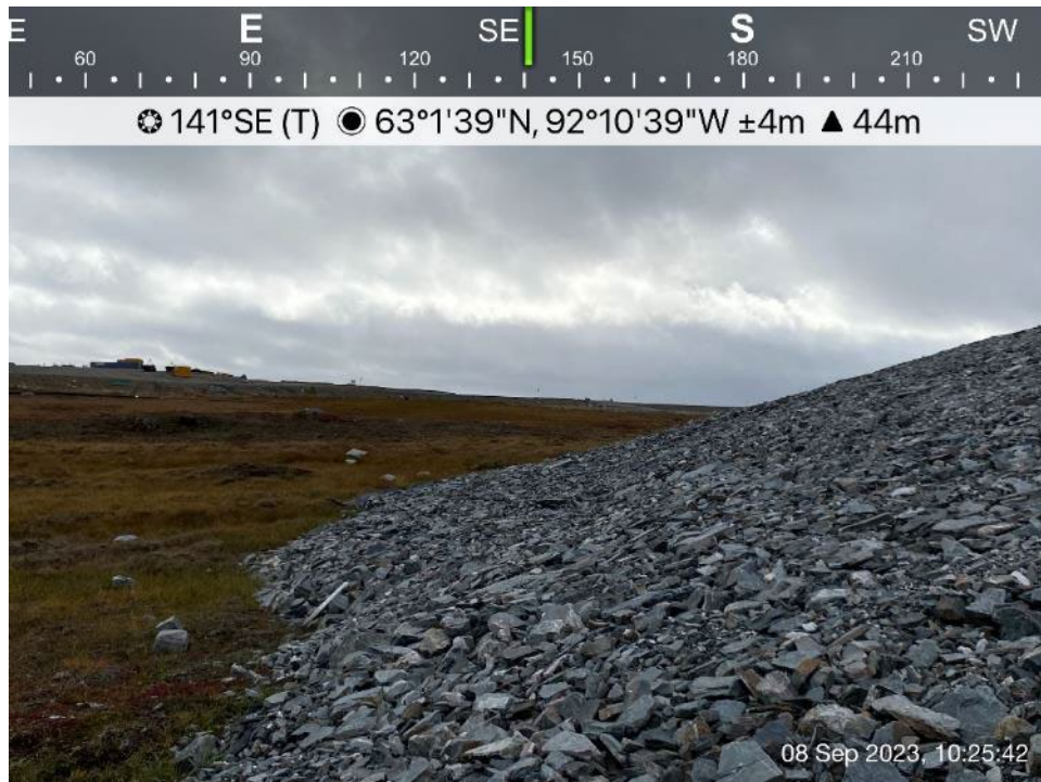
CP2 Thermal Berm - Photo 6: CP2 Thermal Berm - downstream slide slope.
