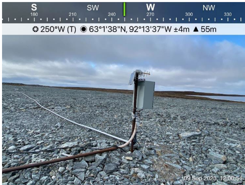
CP4 Thermal Berm - Photo 6: CP4 Thermal Berm - Looking west, GTCs data collection system.
