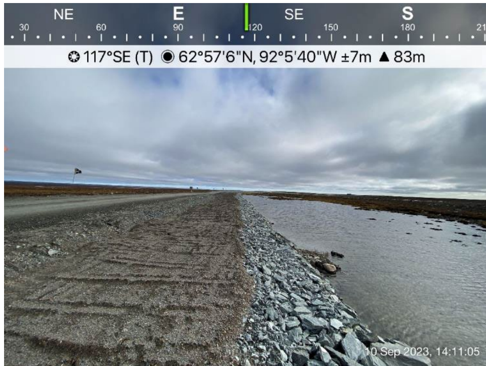
AWAR Road/Culvert - Photo 48: KM 19 - No culvert installed, ponded water upstream, no sign of overflow.
