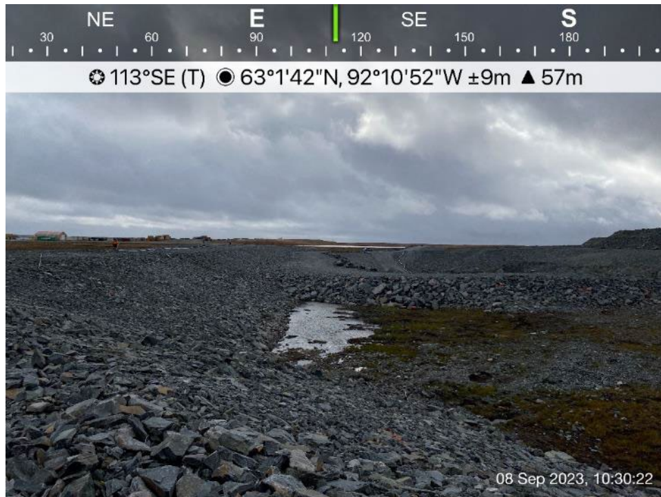
CP2 Thermal Berm - Photo 8: CP2 Thermal Berm - surface ponding observed against upstream toe of CP2 Thermal Berm.
