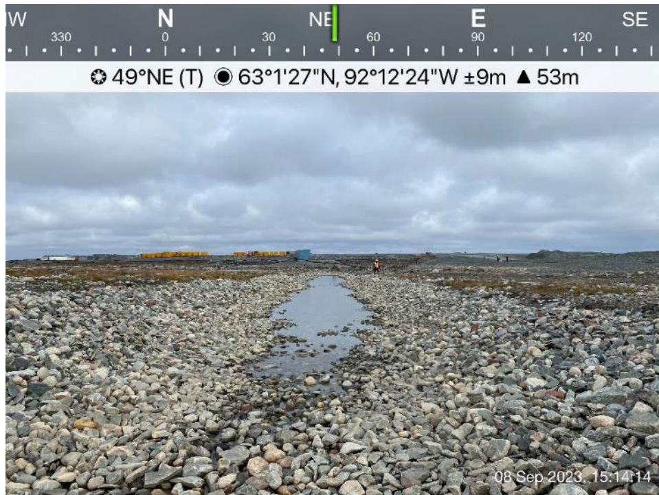
Channel 5 - Photo 10: Channel 5 - Middle section of Channel 5, ponded water observed due to thaw subsidence, looking northeast.
