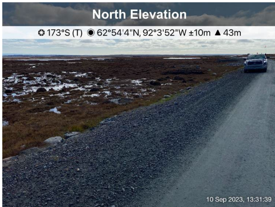
AWAR Road/Culvert - Photo 34: KM 12.6 - No culvert installed, poor drainage condition, no sign of water flow.
