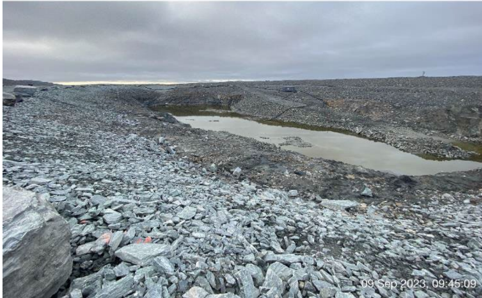
CP3 - Photo 1: CP3 - Small amount of water stored in CP3, bedrock slopes with fractured rock, no stability concern.
