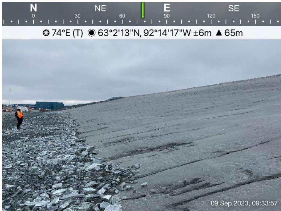
TSF - Photo 3: TSF - Cell 1 north slope surface erosion.
