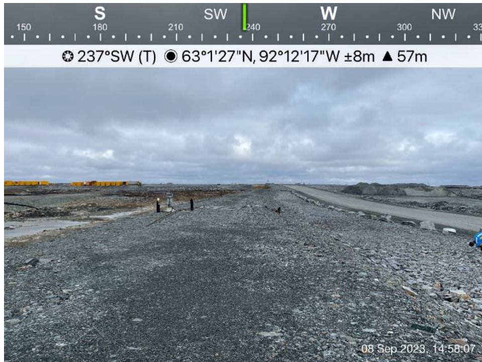
CP5 - Photo 3: Dike D-CP5 - looking southwest, dike downstream side slope and crest.
