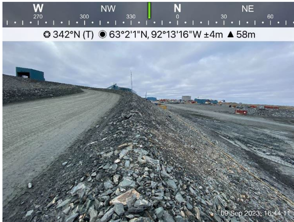
Crusher Pad - Photo 2: Crusher pad ramp and side slope - Overview, looking north.
