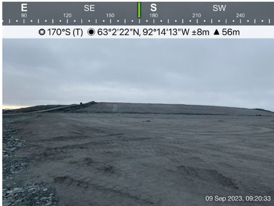
TSF - Photo 1: TSF - Overview of TSF Cell 2 and north slope of Cell 1.
