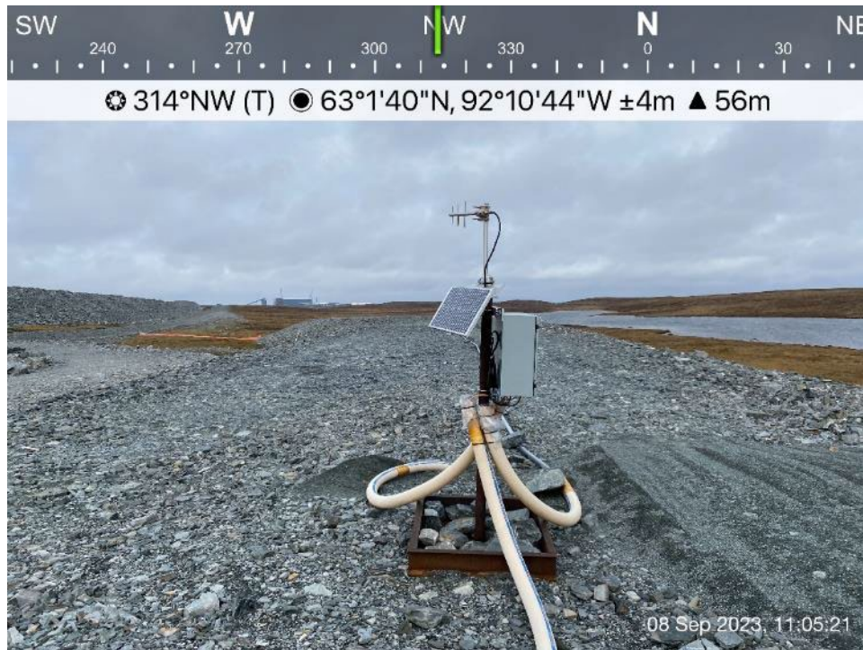
CP2 Thermal Berm - Photo 17: CP2 Thermal Berm - GTC data collection system.
