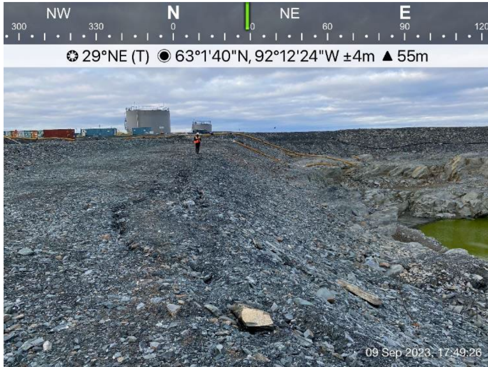
SP1 - Photo 4: SP1 Saline Pond - deformation and cracking in top of overburden protected slope, southwest corner of SP1.
