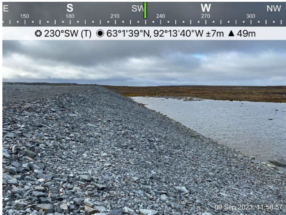
CP4 Thermal Berm - Photo 8: CP4 Thermal Berm - Looking southwest, downstream side slope.
