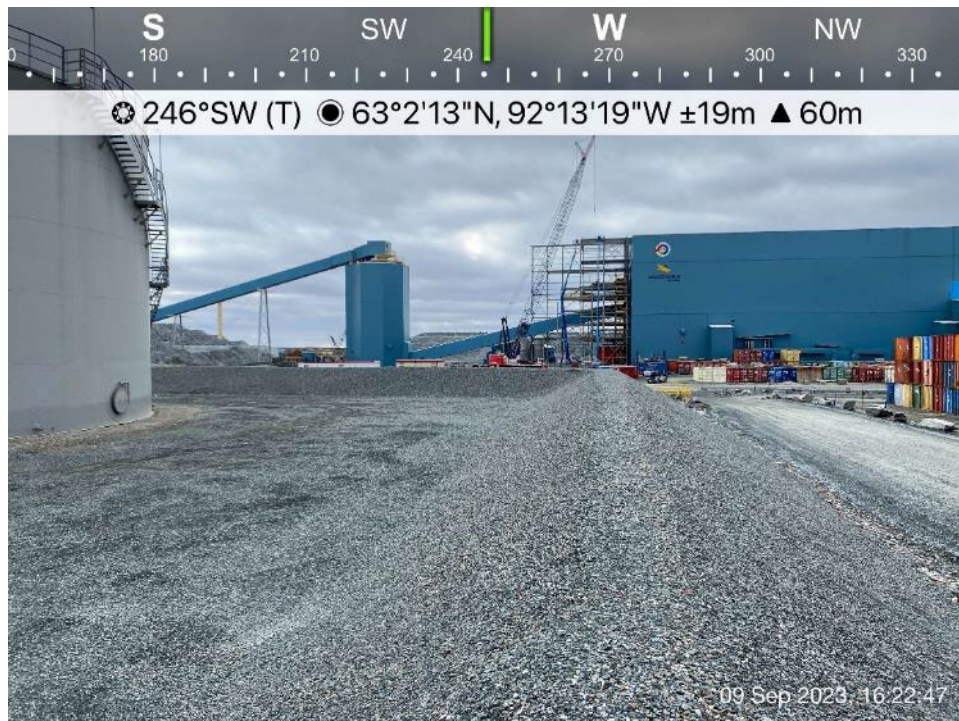
Industrial Fuel Tanks -Photo 24: Industrial Fuel Tanks - north side berm, looking southwest.
