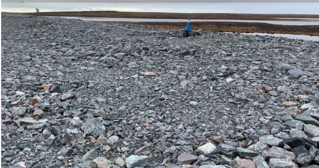
CP3 - Photo 5: CP3 Thermal Berm - Settlement observed on the crest of CP3 Thermal Berm due to thaw settlement.
