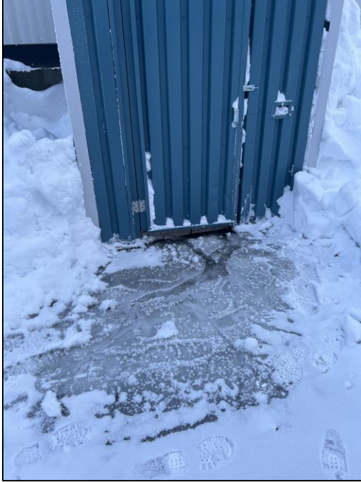
Photo 1: Sewage spill location.
