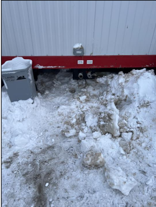
Photo 1: Sewage spill location.
