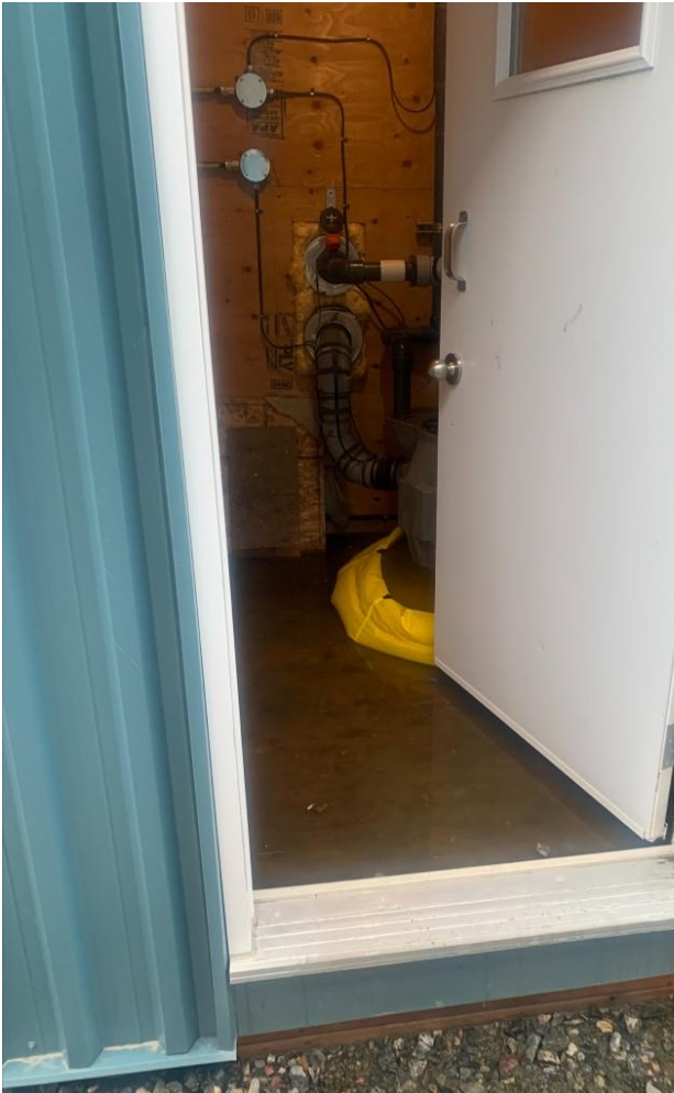
Photos 1 and 2: Sewage spill location.
