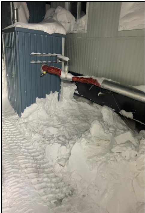
Photo 3: Spill location post remediation.
