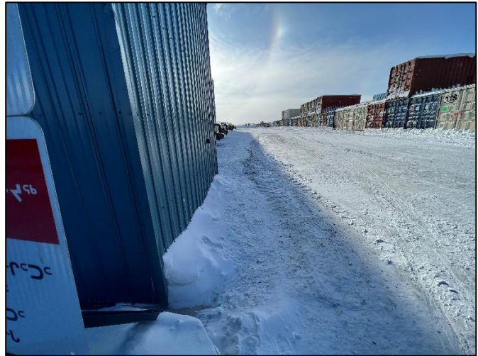
Photo 2: Sewage spill post remediation.
