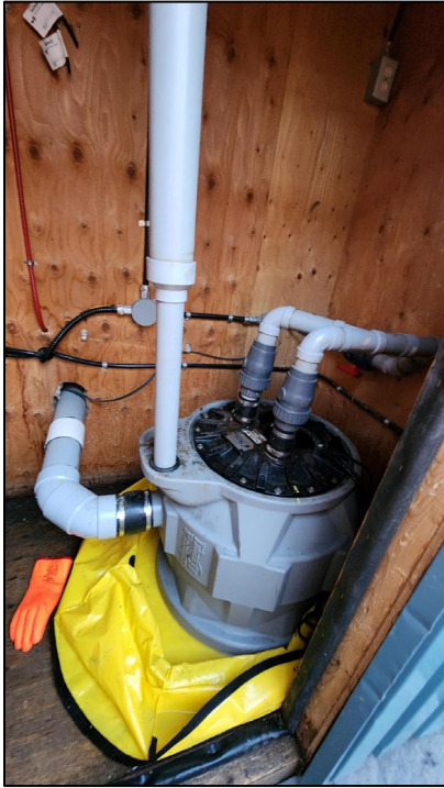
Photo 1: Sewage spill location.
