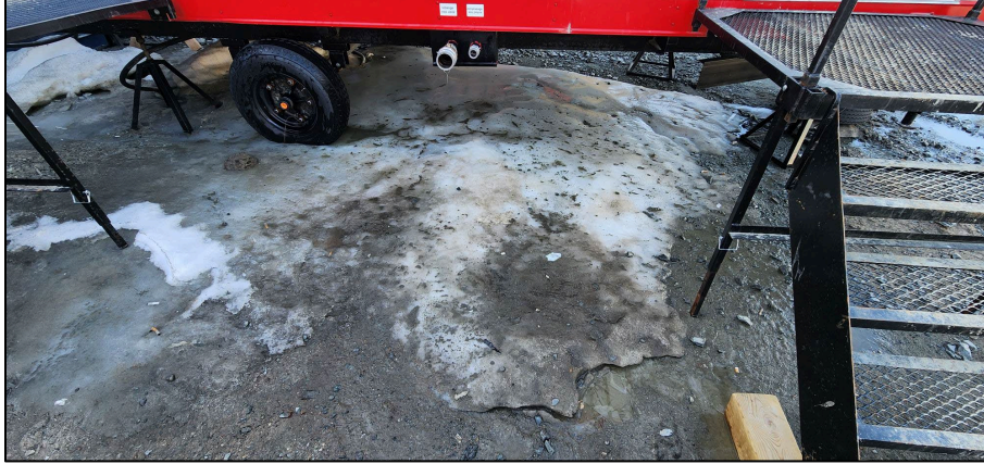
Photos 1: Sewage spill location.
