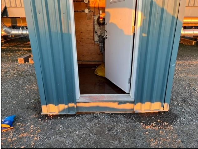
Photos 1: Sewage spill location.
