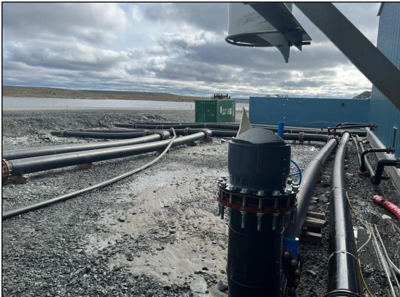
Photo 2: Broken segment of PVC pipe, facing southeast.
