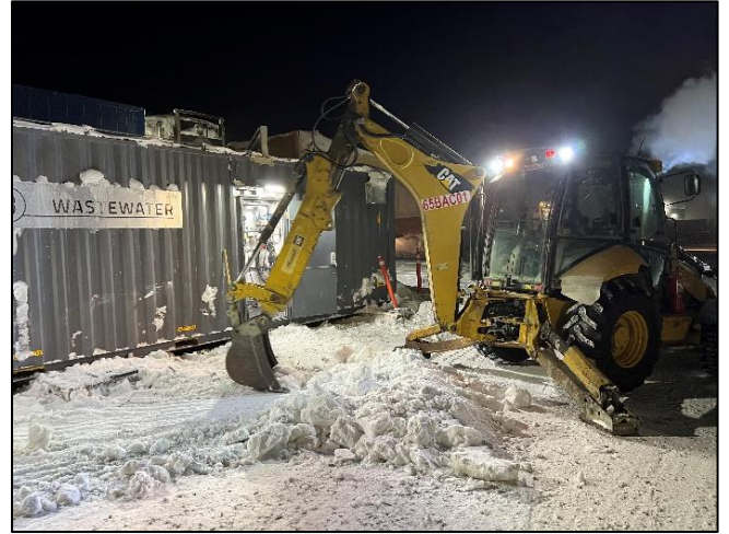
Photo 2: Spill remediation efforts.
