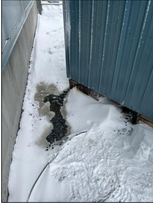
Photo 1: Sewage spill location.
