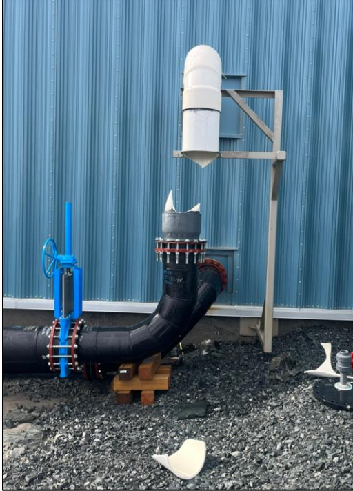
Photo 1: Broken segment of PVC pipe, facing southwest.
