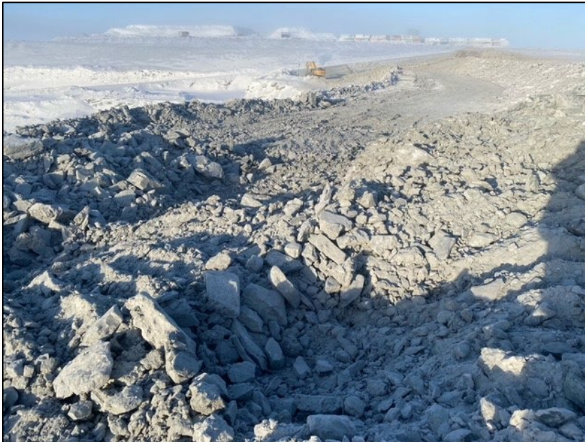
Photo 2: Hydraulic oil spill remediated.
