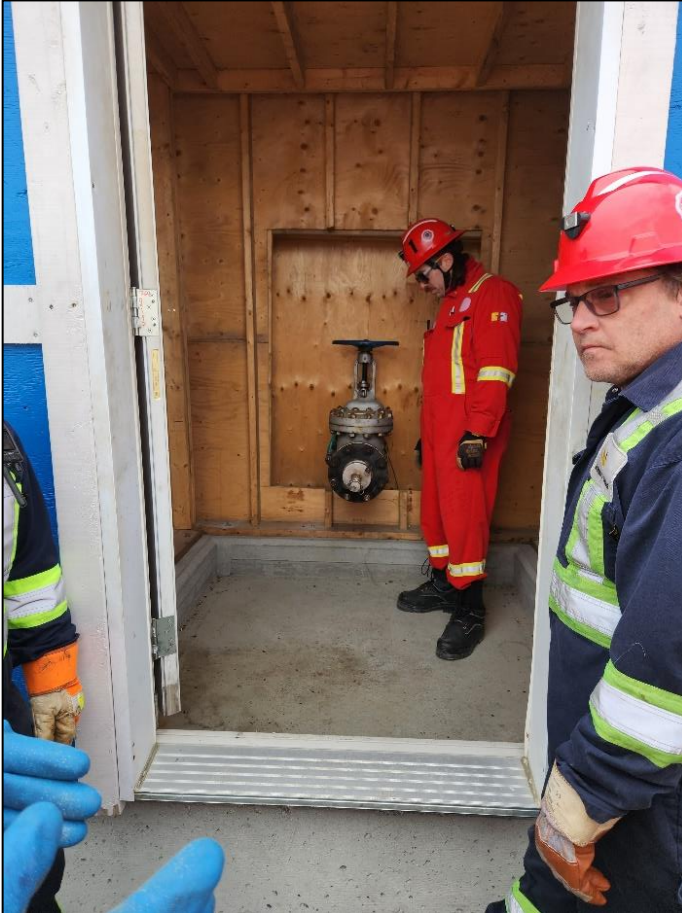
Photo 1: Mock spill scenario location (leak from piping flange).
