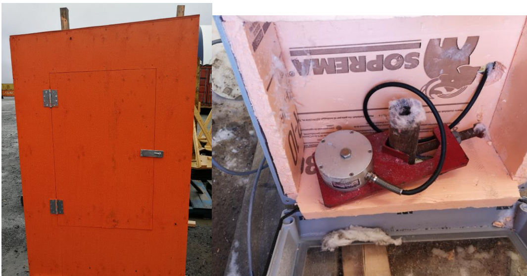
Figure 6. Surface Installation (Shelter & installation inside)
