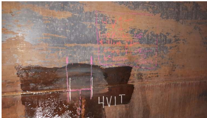
Photo #6: Lack of fusion found T intersection ring level 4 - plate 1 - Top horizontal position
