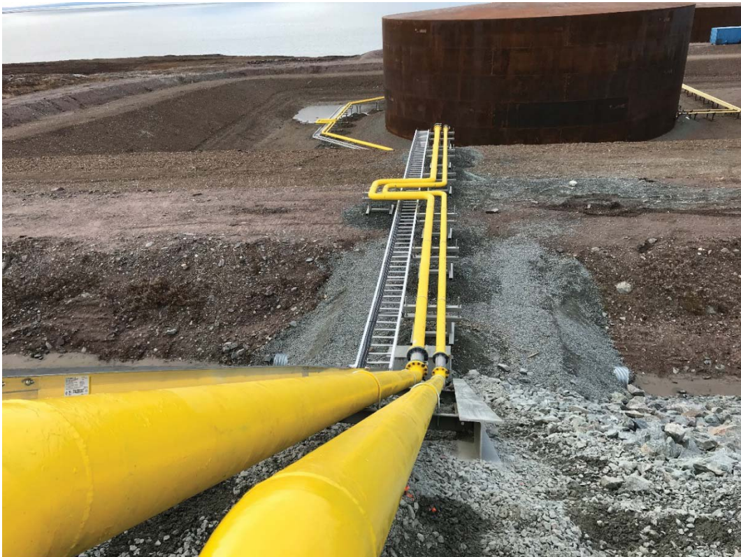
Piping to and from fuel tank
