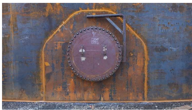
Photo #8: Manway (180 degree)
