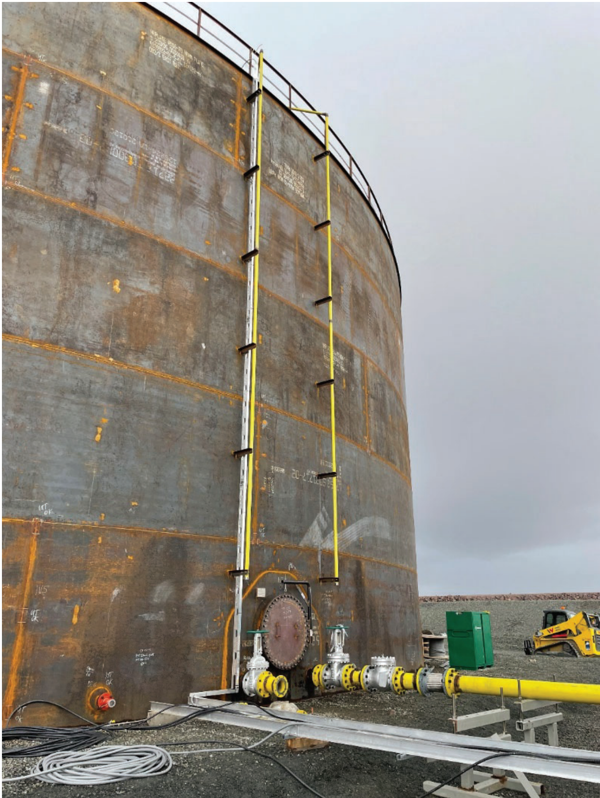
Control cable tray and over pressure valve piping
