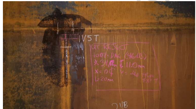
Photo #7: Lack of fusion found T intersection ring level 1 - plate 5 - Top vertical position
