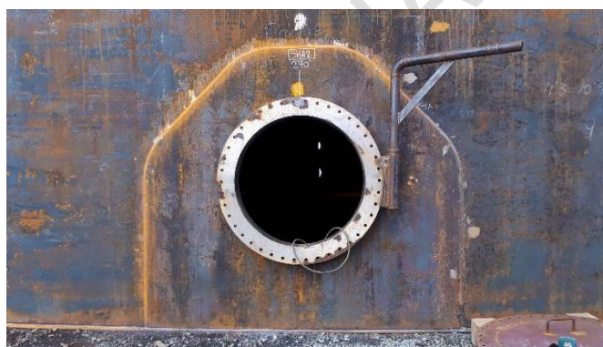
Photo #12: Manway (270 degree)
