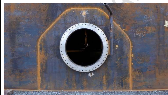
Photo #6: Manway (90 degree)
