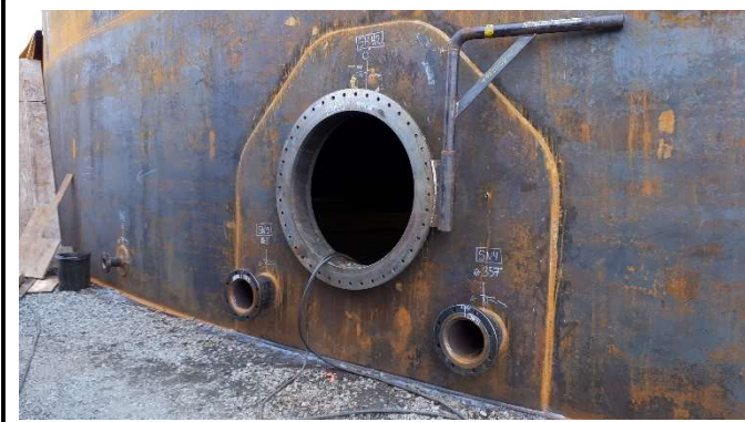
Photo #2: Manway (0 degree) Nozzles SN3 (3degree) & SN4 (357 degree)
