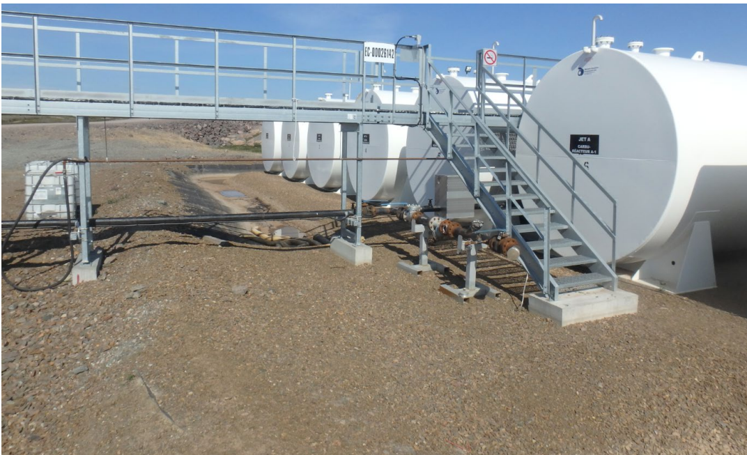
Photo 2. Jet-A Transfer - Connection between shipper transfer hoses and Agnico Eagle permanent pipeline
