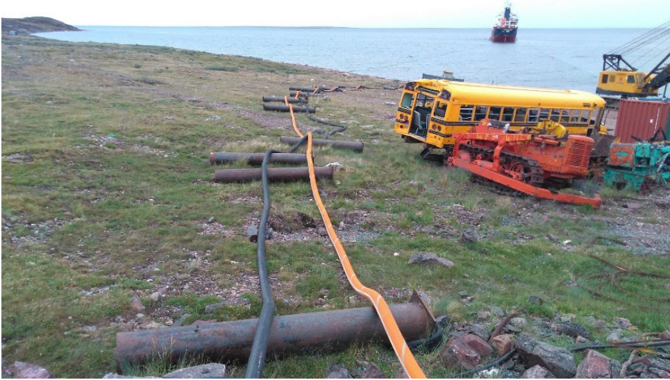
Photo 1. Diesel Transfer - Connection between shipper transfer hoses and Agnico Eagle permanent pipeline
