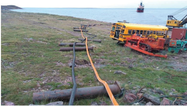
Photo 1: Diesel Transfer - Connection between shipper transfer hoses and Agnico permanent pipeline
