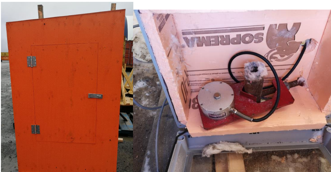
Figure 6. Surface Installation (Shelter & installation inside)
