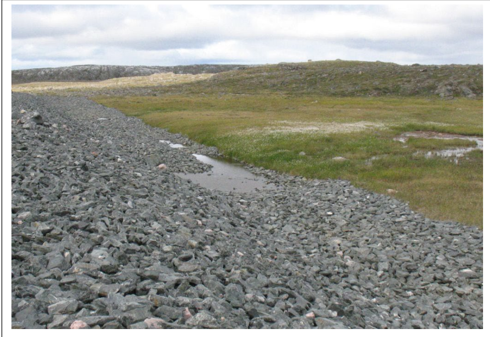
Photo #3 IVR Diversion Ditch. Localized thaw settlement.
