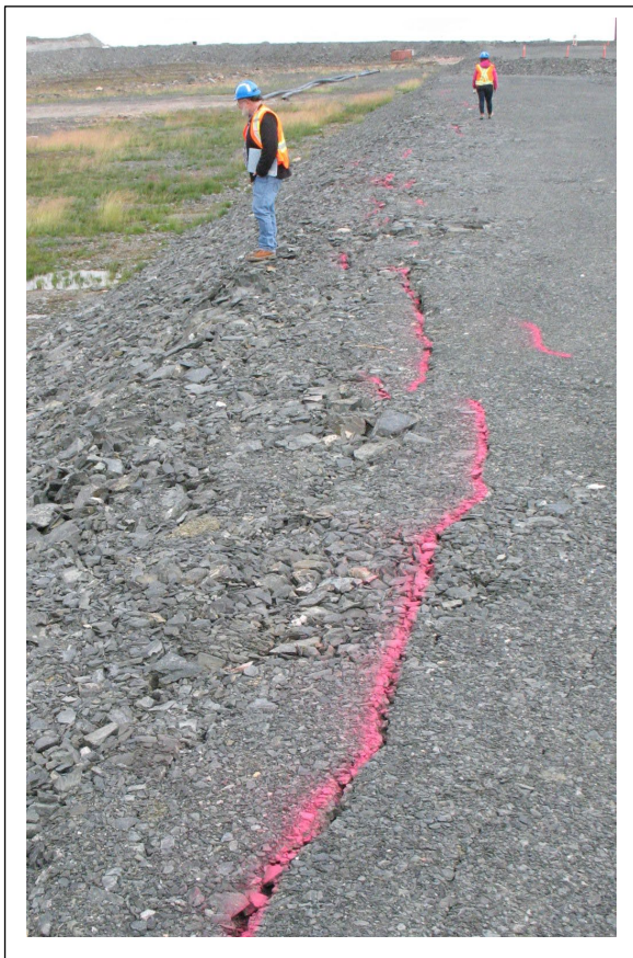
Photo #2 IVR Dike crest. Cracks observed during surveillance.
