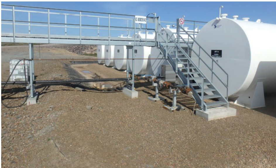
Photo 2: Jet-A Transfer - Connection between shipper transfer hoses and Agnico permanent pipeline
