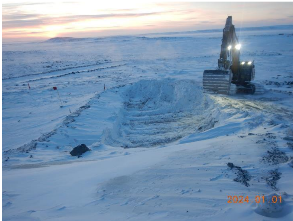
Figure 8. Water Inflow investigation Jan 1, 2024
