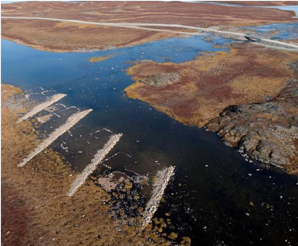
Figure 1. Arctic Grayling spawning pads constructed at Meadowbank all weather road crossing R02.
