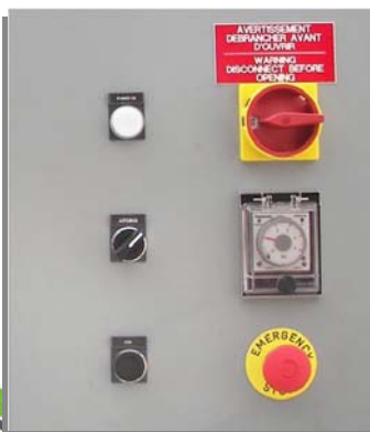
Figure 2 -- Brome Composter Control Panel
