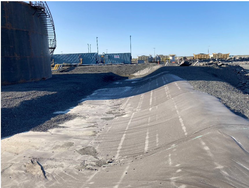
Photograph G3-4 Whale Tail Project Site Tank Farm
