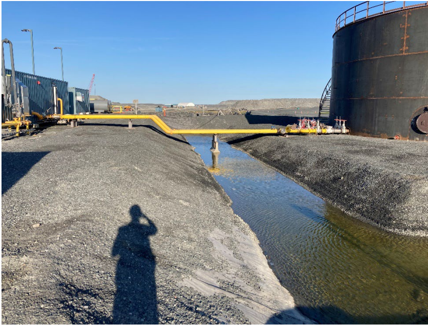
Photograph G3-1 Whale Tail Project Site Tank Farm
