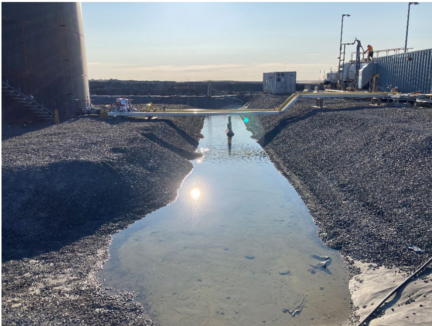
Photograph G3-7 Whale Tail Project Site Tank Farm
