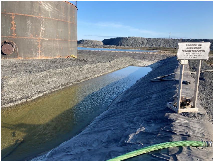
Photograph G3-2 Whale Tail Project Site Tank Farm
