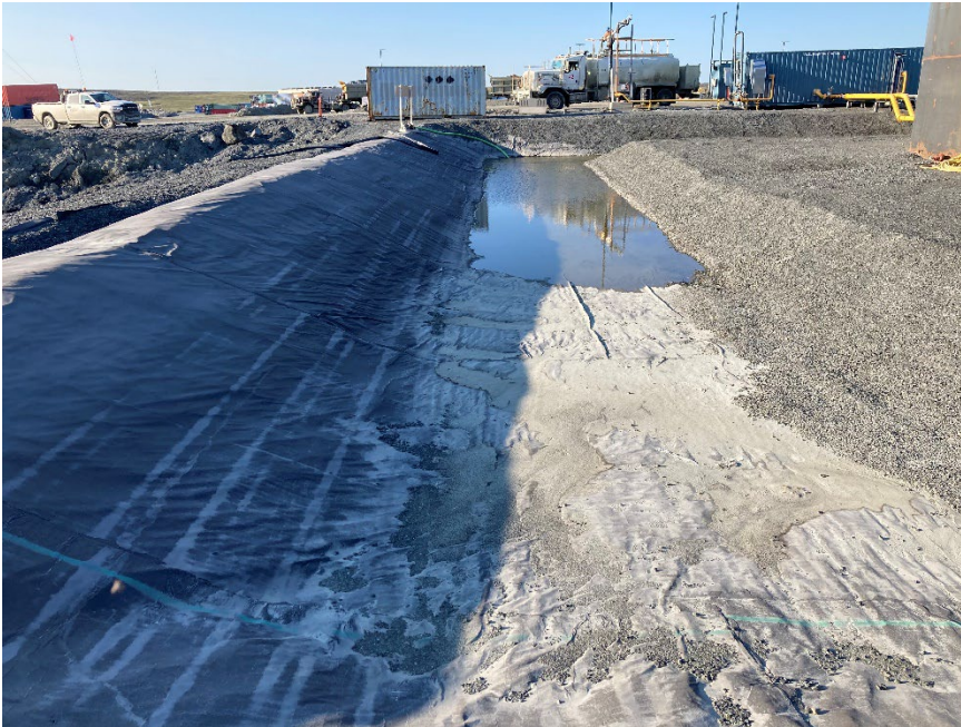
Photograph G3-6 Whale Tail Project Site Tank Farm
