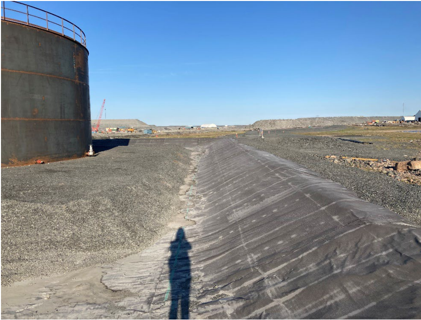
Photograph G3-5 Whale Tail Project Site Tank Farm
