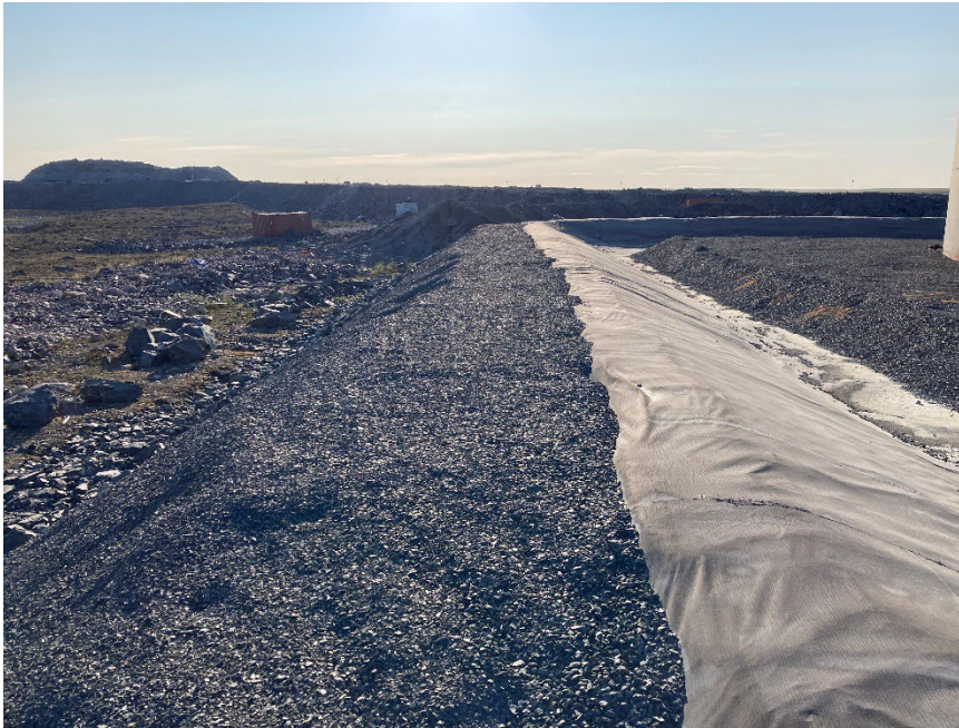
Photograph G3-3 Whale Tail Project Site Tank Farm
