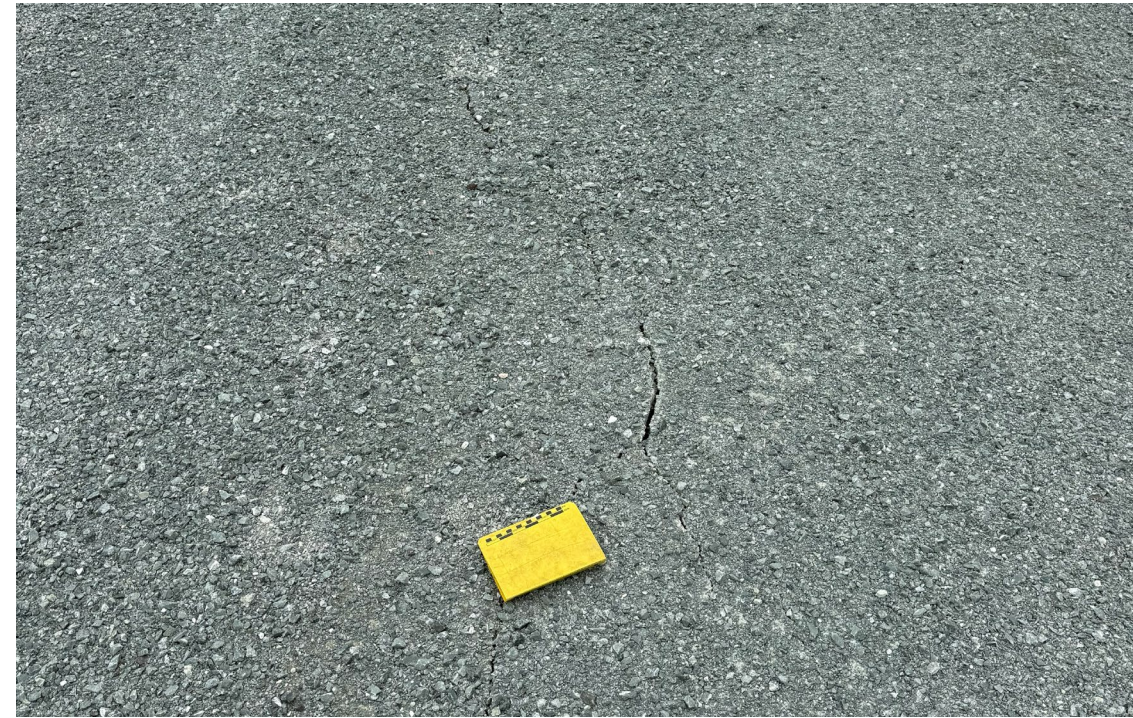
Photo 26: Airstrip shoulder tension cracking
