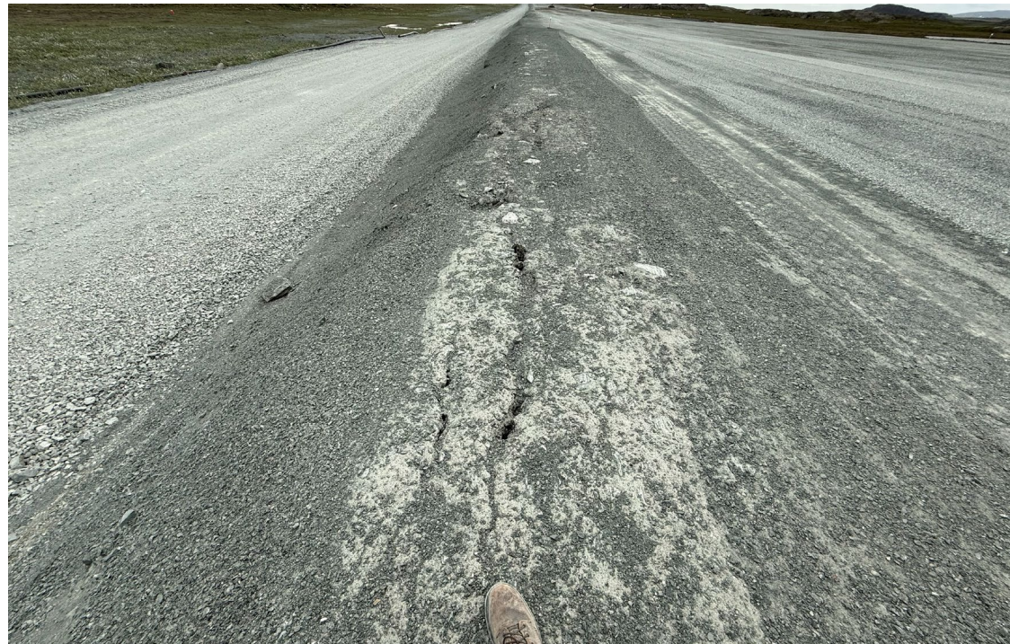
Photo 27: Airstrip shoulder tension cracking at the edge
