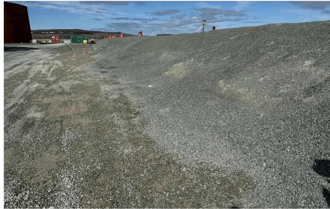
Photo 6: Multi-tank farm (20M liter) east berm
