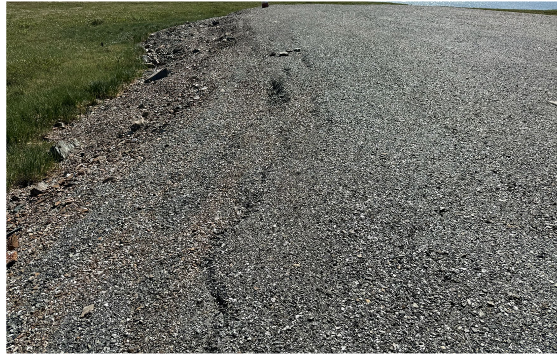
Photo 10: Tension cracking along shoulder of Boston Airstrip
