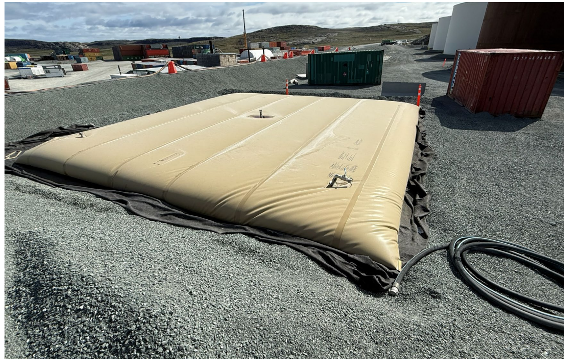
Photo 7: Multi-tank farm (20M liter) – Additional fuel bladder located within the tank farm
