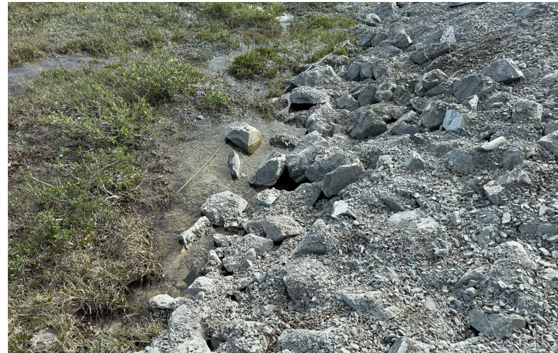
Photo 24: Helicopter Pad downstream flowing water emanating from toe
