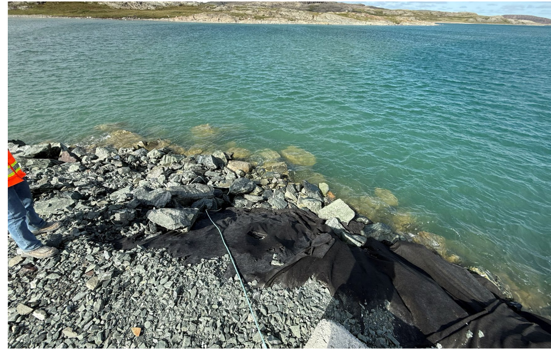
Photo 2: Exposed geotextile on the marine outfall berm
