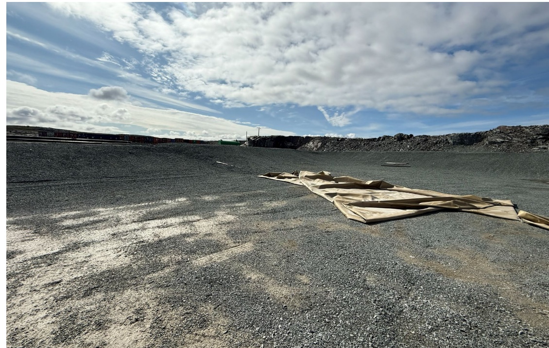
Photo 8: Quarry 1 (50M liter) tank farm
