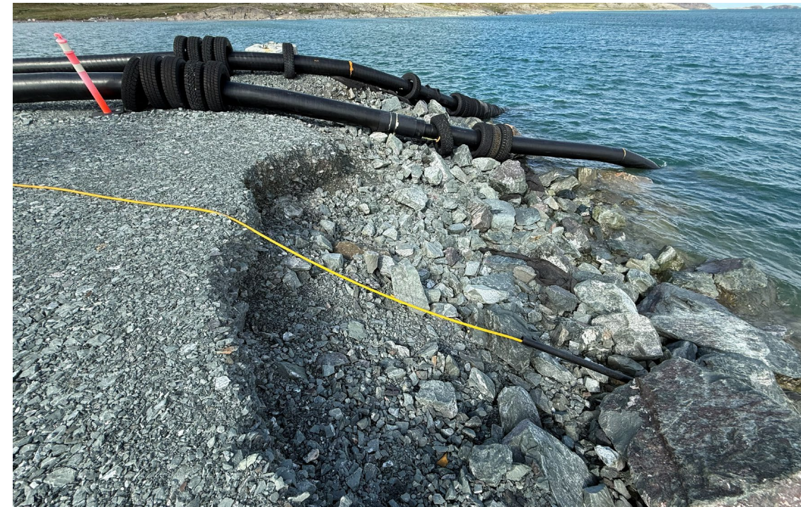
Photo 4: Short vertical face at end of marine outfall berm due to wave erosion
