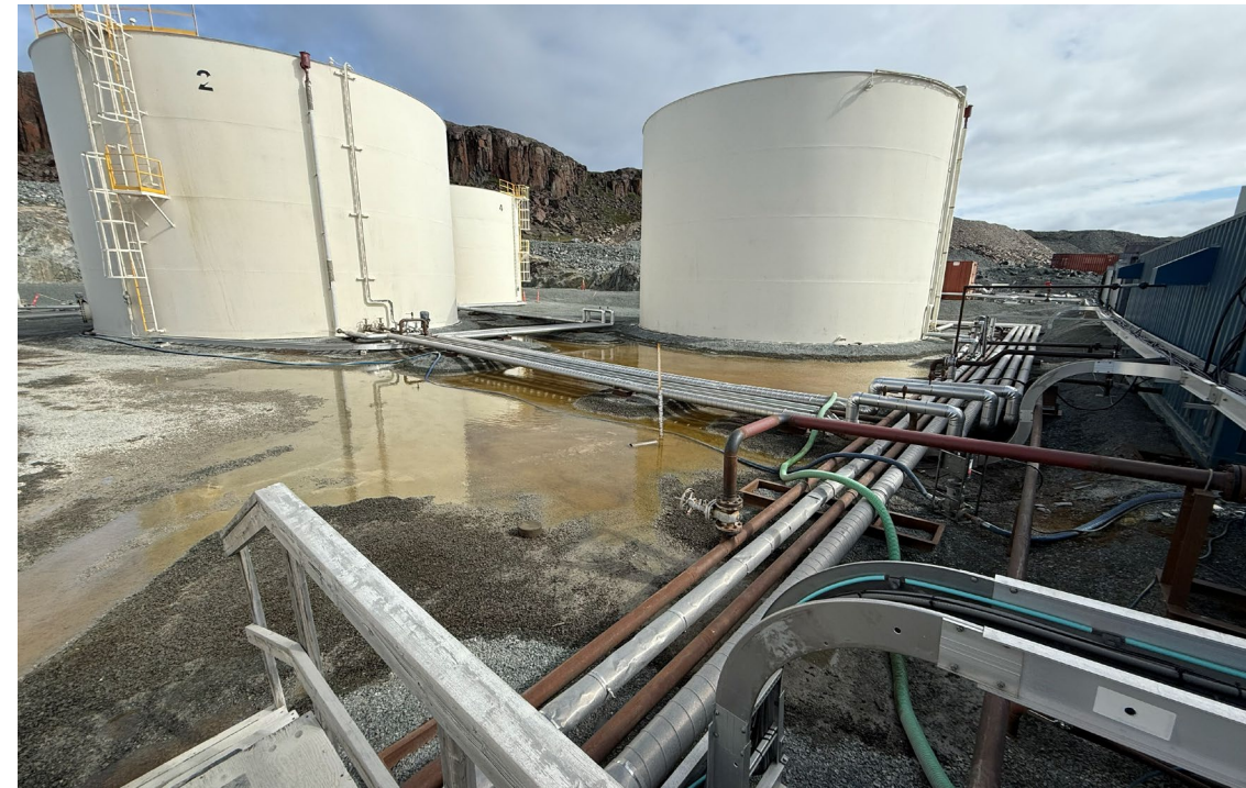
Photo 20: Doris tank farm water accumulation
