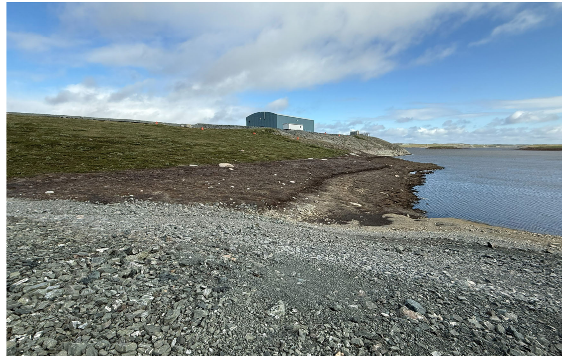
Photo 4: North Dam Upstream Toe Tundra Die-Back
