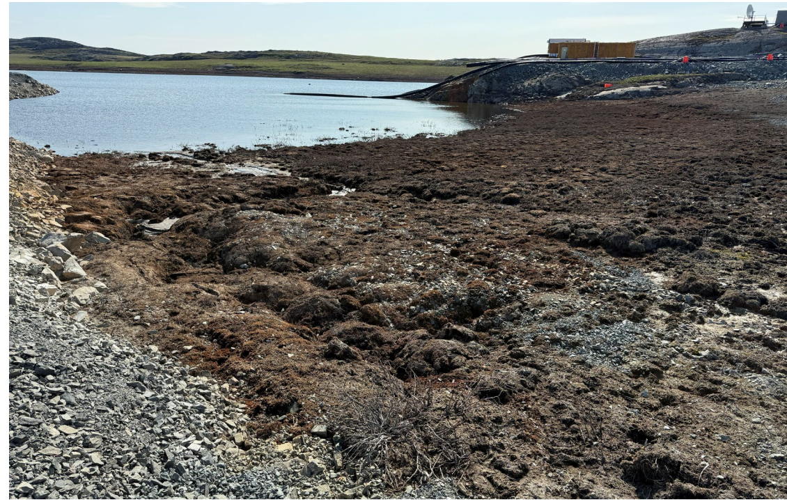
Photo 34: Shoreline Degradation near the previous Reclaim Jetty.
