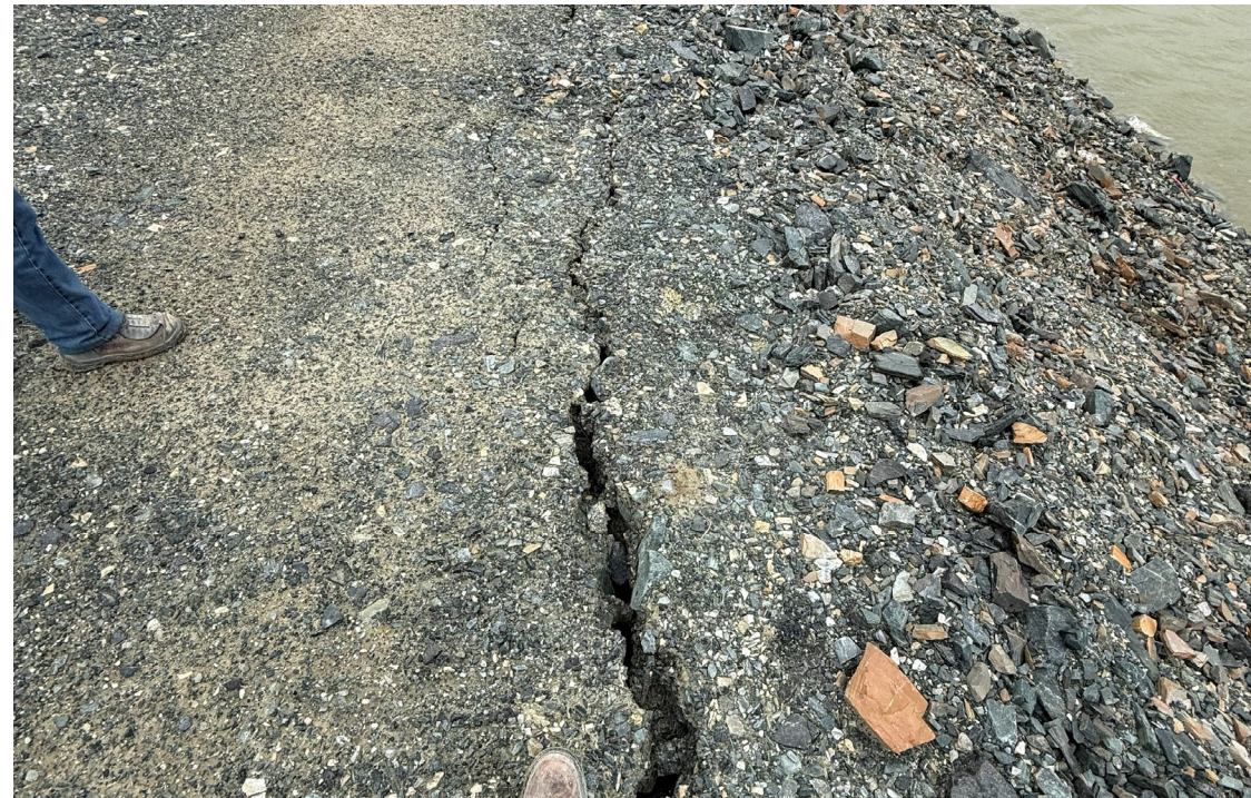
Photo 19: Interim Dike Upstream Crest Tension Cracking
