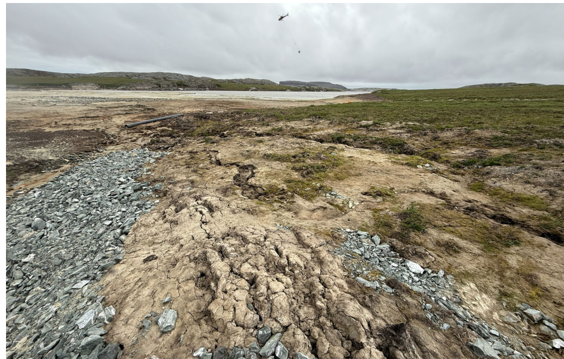
Photo 23: Interim Dike Water Elevation Control Channel shoulder, erosion near outlet
