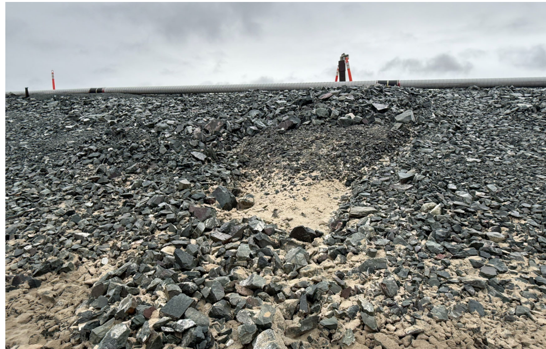
Photo 13: South Dam Downstream Face Excavator Mark
